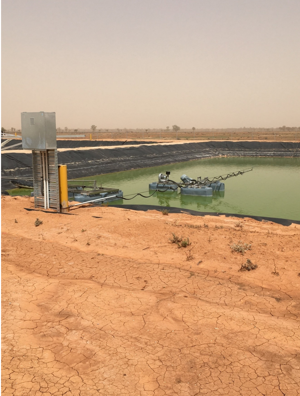
(Photo 15: Wastewater Treatment Pond, Aerator Cables, Anchor Points and fencing.)
