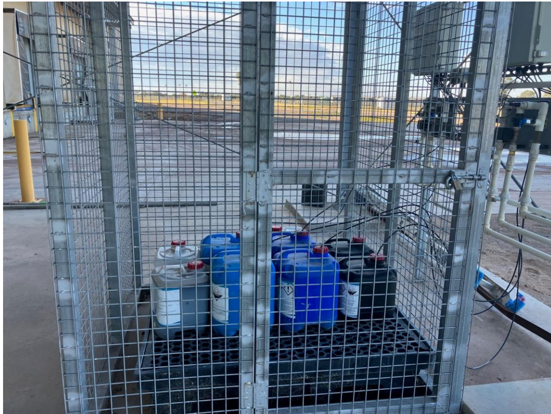
Figure 9: Water dosing chemical stored on a bunding
