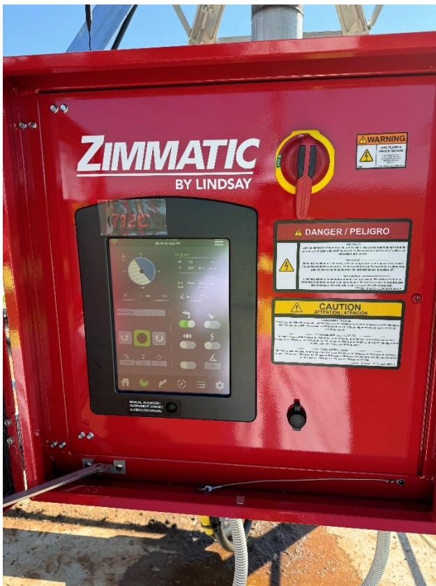
Figure 20: Center Pivot Control Panel
