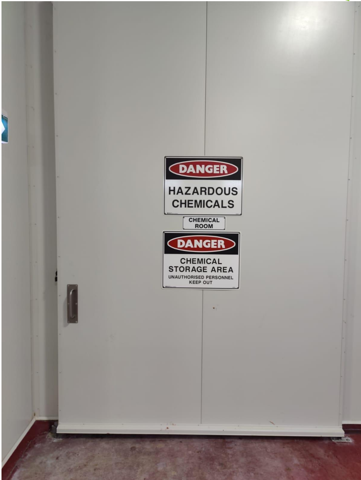
Figure 14: Chemical Room Signage (b)
