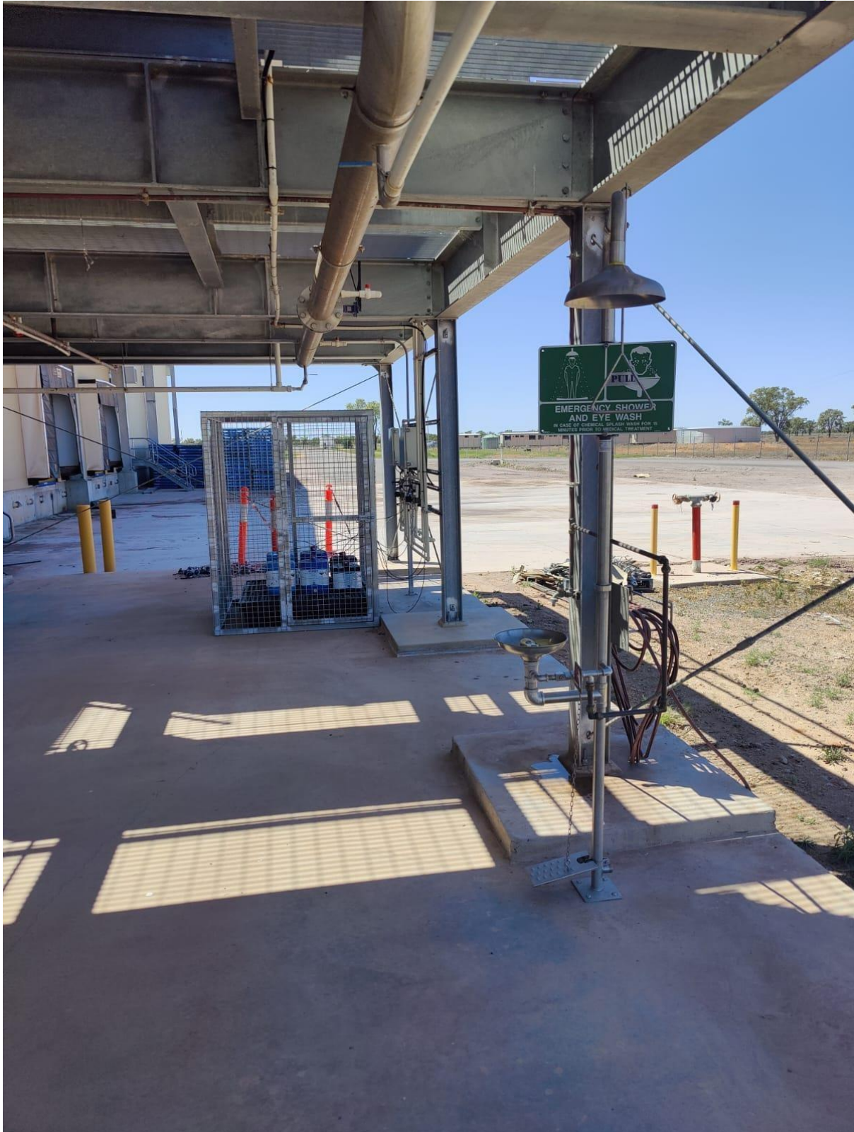
Figure 12: Water dosing chemical stored on a bunding
