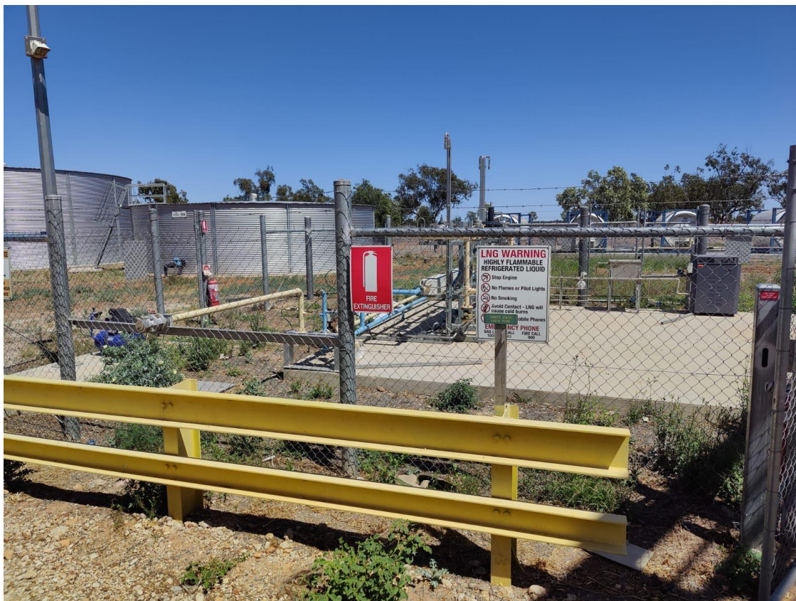
Figure 11: Safety Signs for LPG filling area
