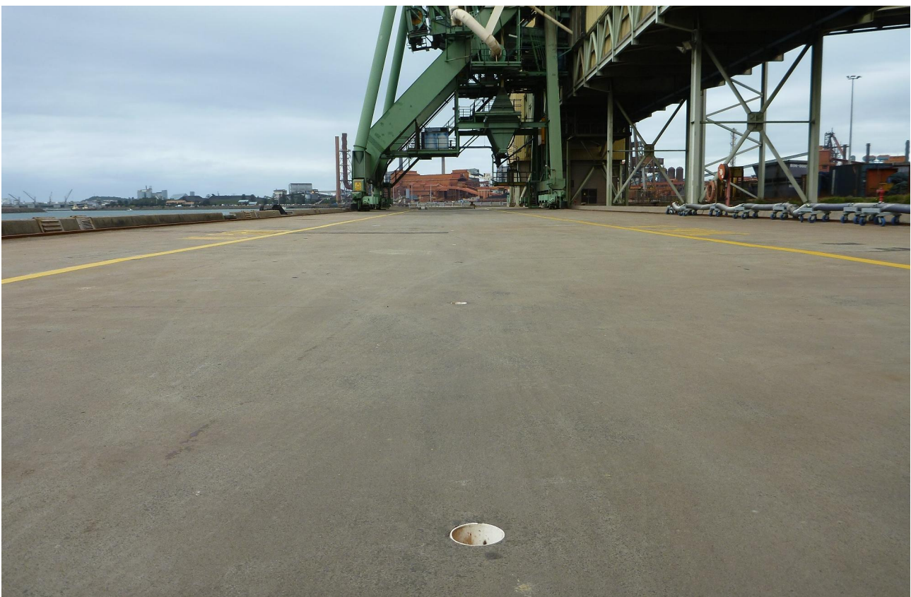
Figure 2-7 Existing Drainage on Berth 104 (Looking South)
