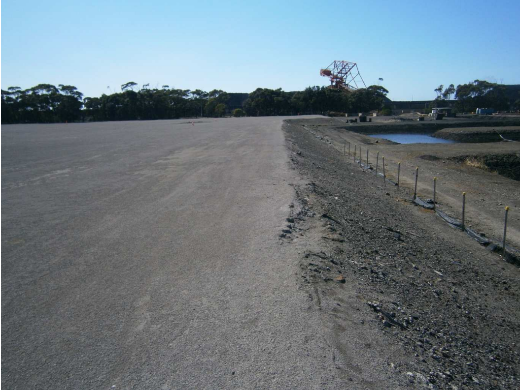
Photo 9: Looking east across the southern boundary of Zone 2 showing raised fill terrain
