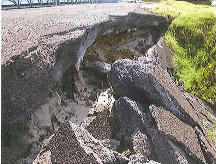
Plate 4. Allotment 5 slumping of fill material, looking north.
