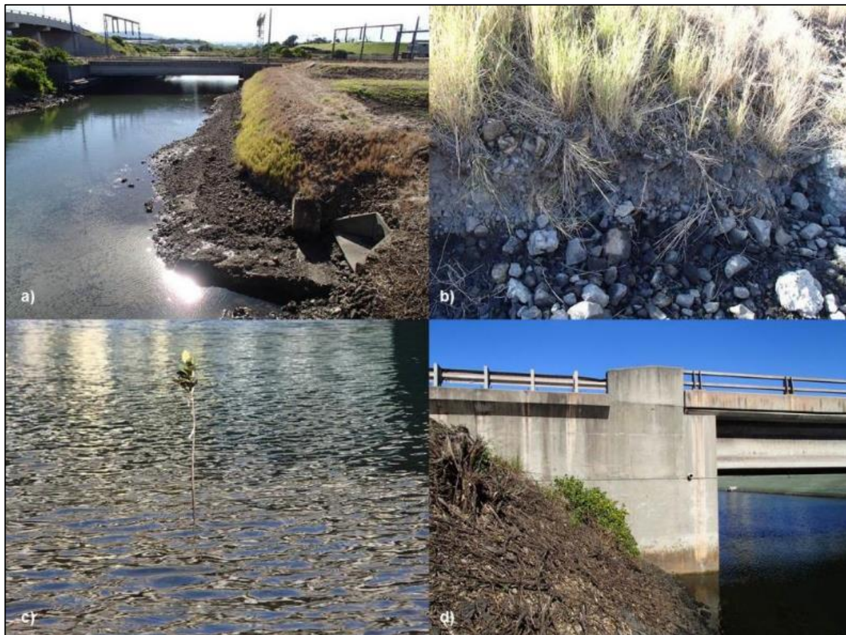
Figure 3-15 Unconsolidated rock substrata (a), undercutting and erosion of the existing earthworks (b), grey mangrove ( Avicennia marina ) (c) and bitou bush ( Chrysanthemoides monilifera ) (d) recorded at Site 3
