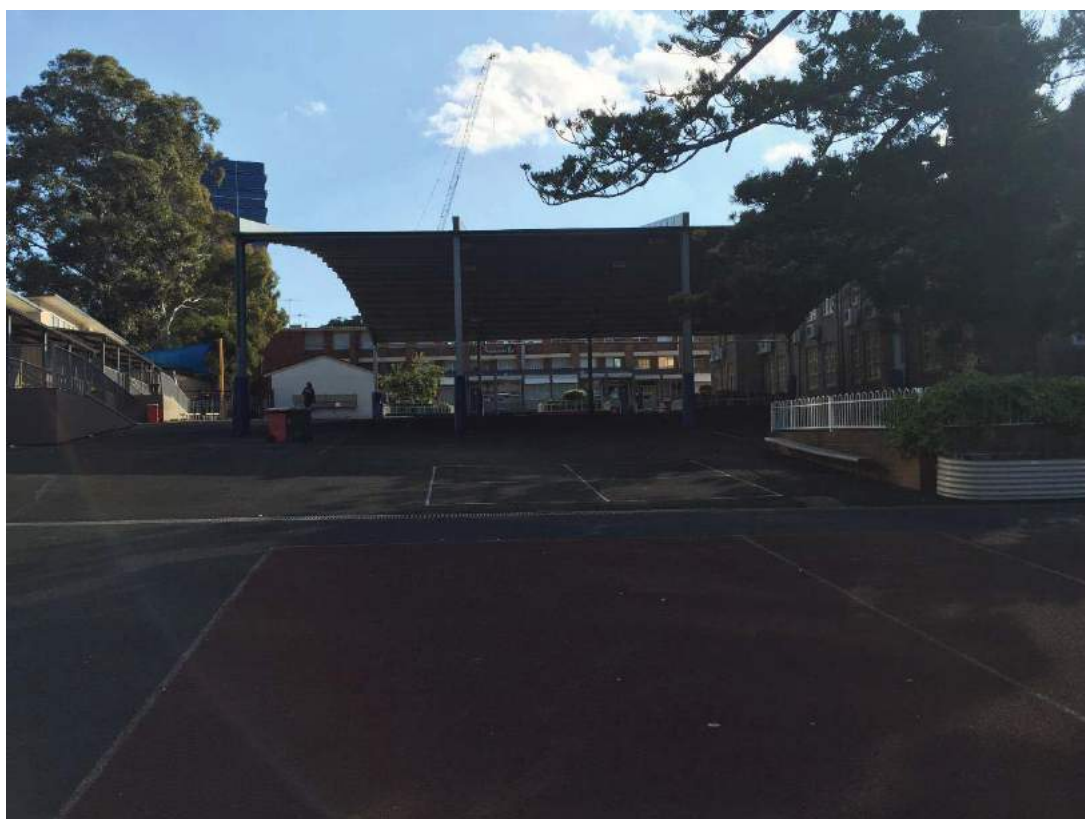
Photograph 11: Parramatta Public School playground with soft bitumen on surface, looking west.
