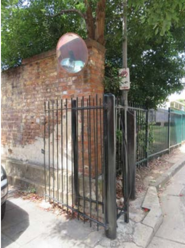
Figure 3.9 Section of the heritage convict brick wall at the western end of the north boundary of the site. The wall shows signs of reconstruction including the concrete reinforcement of the lower northern skin. (GML 2016)
