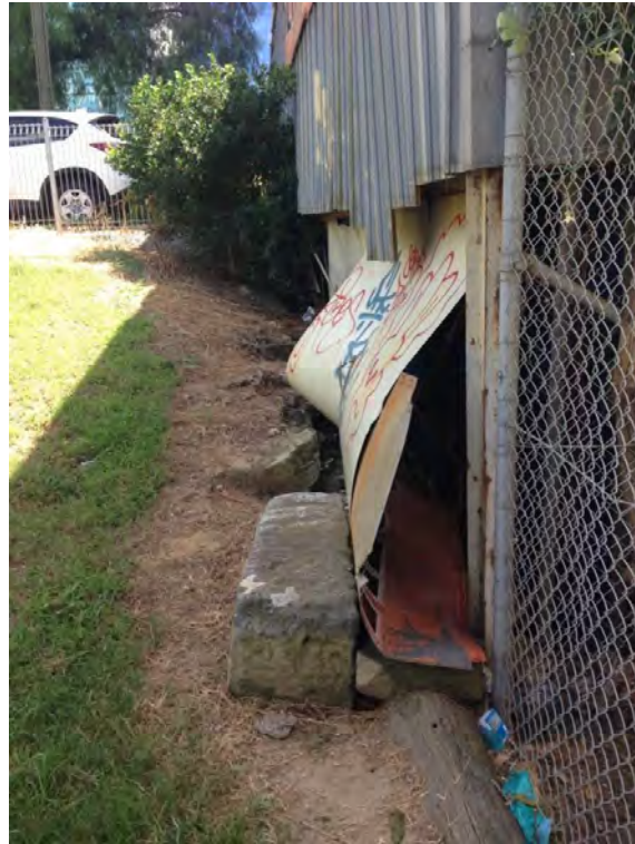
Figure 3.64 Loose sandstone blocks at the eastern end of the convict barracks wall.
