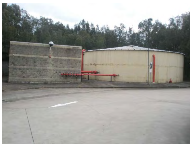
Plate 3: View of the fire water tank and diesel pump room
