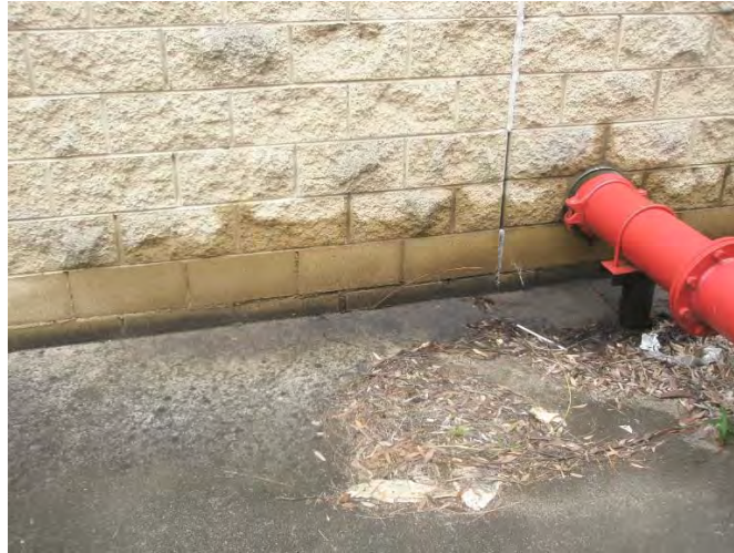
Plate 4: View of diesel pump room with staining on external wall
