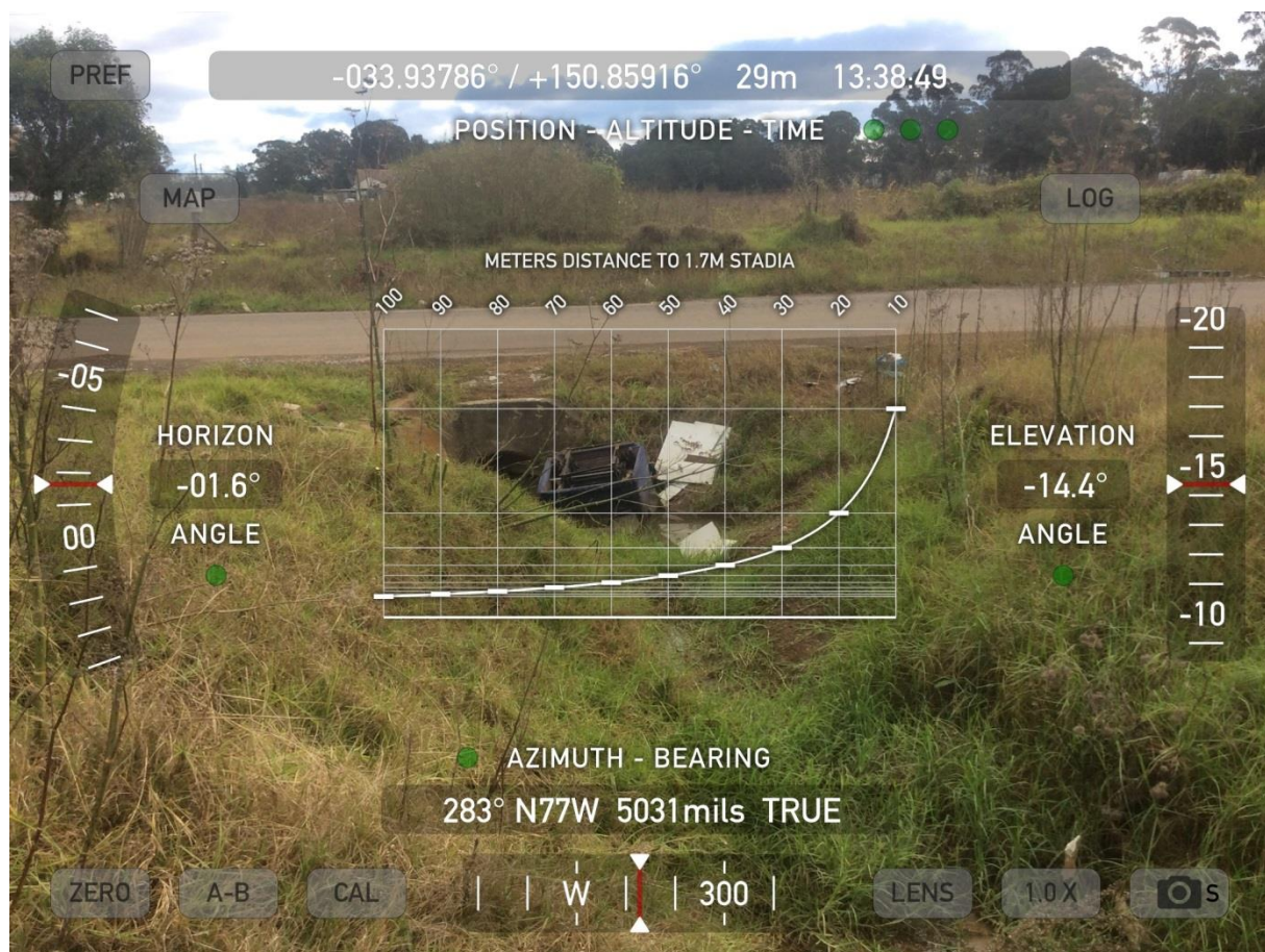
Photo 1 Stormwater headwall and open drainage channel running off Kookaburra Road
