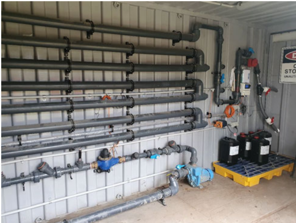
Photograph 9 – (8 Styles St) Dosage unit for water treatment of collected water stored in dam.
