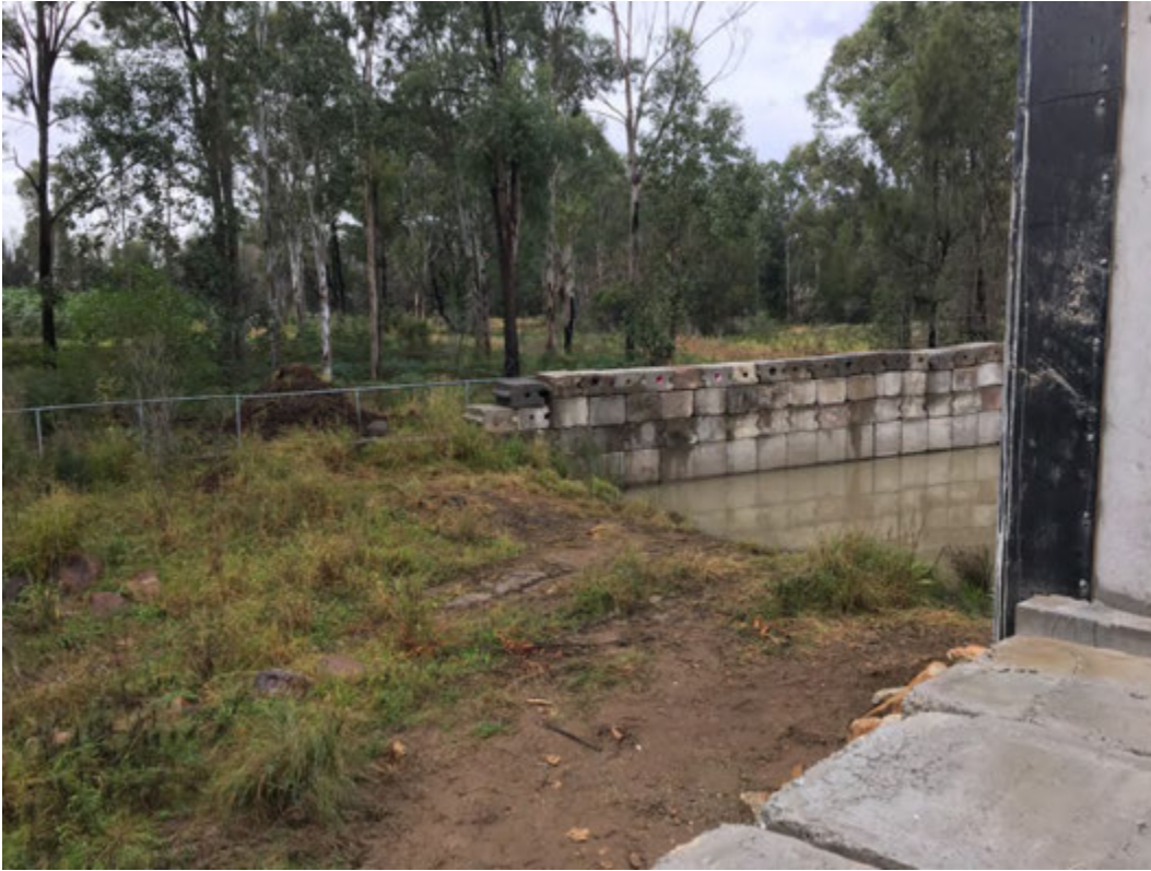
Photograph B.7 Sedimentation basin at eastern boundary of the site - facing east (June 2018). Construction works to line the area to commence in January 2019
