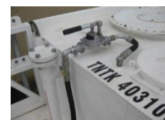
"Typical" Dewatering pump
