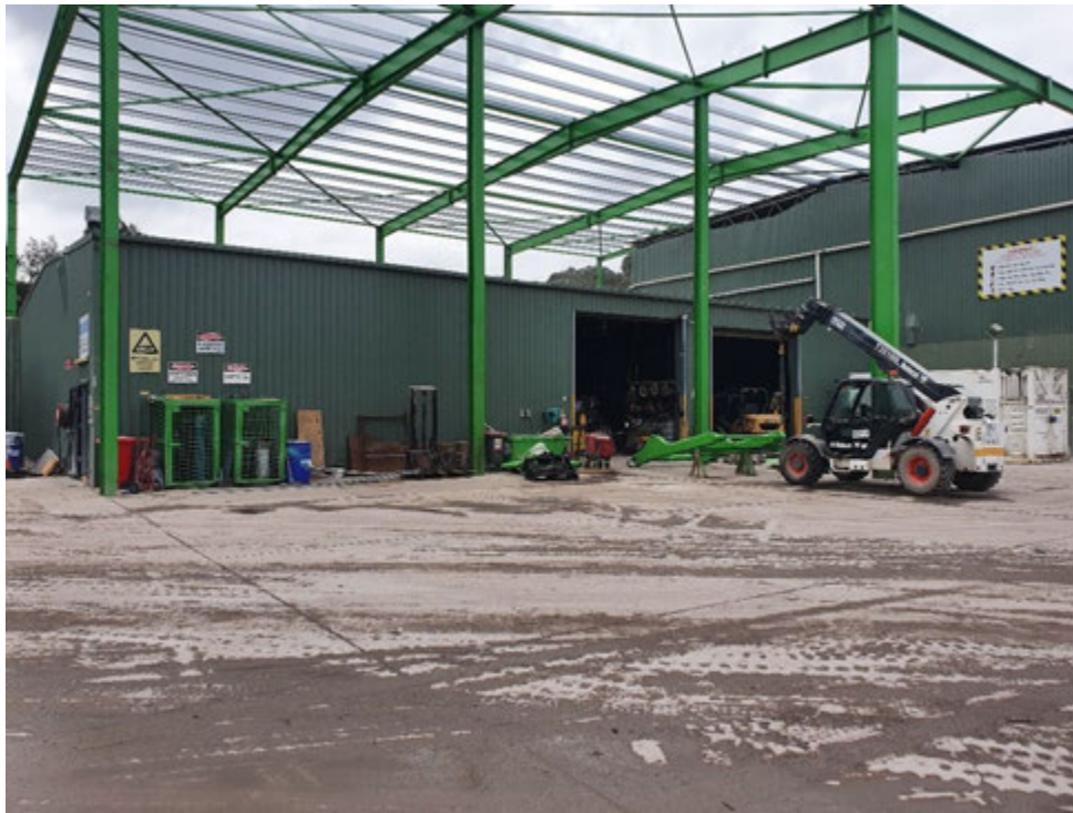
Photograph 3 – (8 Styles St) Workshop area of CWS main processing plant. A larger workshop was under construction at the time of the Site inspection 14 th October 2020.
