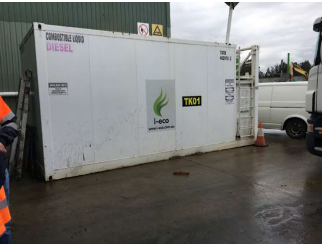
Photograph B.3 Bunded diesel above ground storage unit on slab (June 2018)
