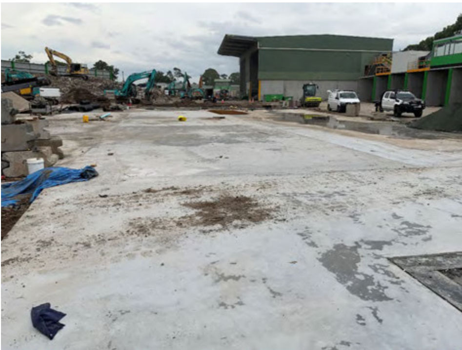
Photograph B.11 Concrete slab laid in previously unsealed area. Temporary concrete storage now on sealed areas of the site (December 2018)
