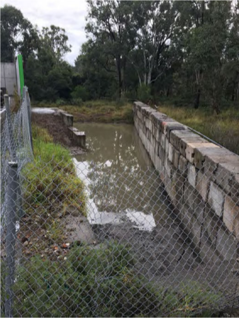
Photograph B.12 Water detention area looking north on eastern boundary of site (June 2018). Construction works to line the area to commence in January 2019.
