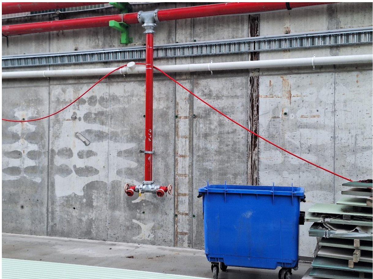
Plate 4: Hydrants on the northern side of the material processing shed
