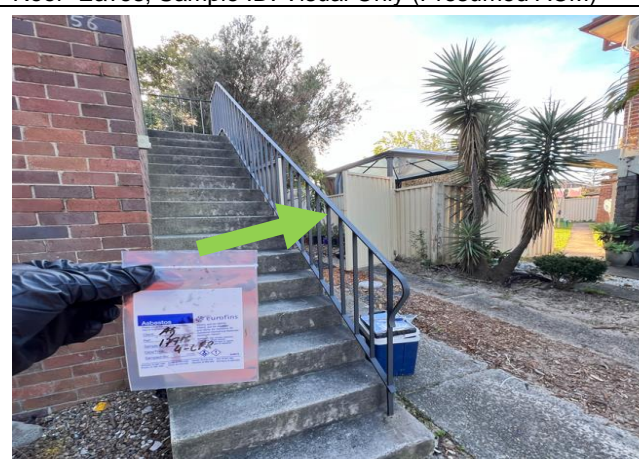
Photograph 4 (20.06.24): Representative photo of dark grey paint system, external, northern side staircase handrail, Sample ID: 4-L2 (0.07 % w/w)
