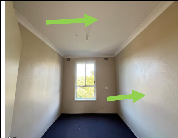
Photograph 19 (20.06.24): Representative photo of yellow paint system (walls) and white paint system (ceiling) and white coloured plasterboard (ceiling), internal Room 2 Sample ID: Lead - Same as 4- LP 8 (< 0.01 % w/w) and Asbestos – Same as A1 (NAD).
