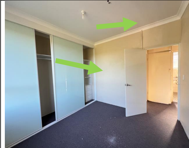
Photograph 21 (20.06.24): Representative photo of yellow paint system (walls), white paint system (ceiling) and white coloured plasterboard (ceiling), internal Room 4, Sample ID: Lead - Same as 4- LP 8 (< 0.01 % w/w) and Asbestos – Same as A1 (NAD).
