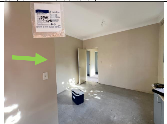
Photograph 12 (20.06.24): Representative photo of yellow paint system, internal kitchen walls on all four walls, Sample ID: 4-LP 8 (< 0.01 % w/w).
