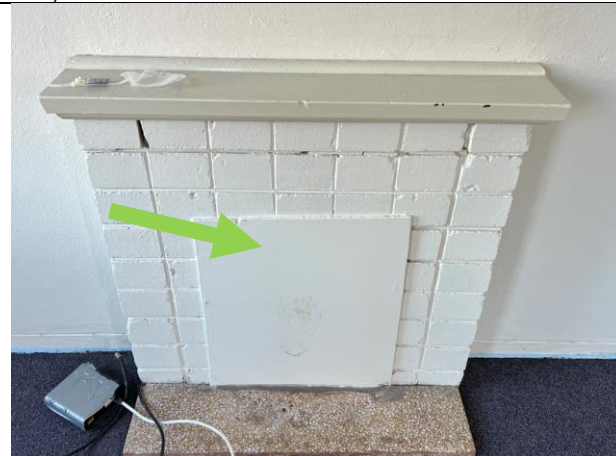
Photograph 18 (20.06.24): Representative photo of yellow coloured plasterboard, internal Room 1 on the fireplace cover, Sample ID: A5 (NAD).
