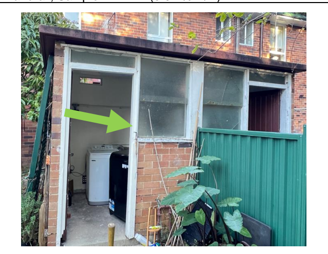
Photograph 6 (20.06.24): Representative photo of white paint system, external backyard laundry shed door frame, Sample ID: 4-LP4 (0.09 % w/w)
