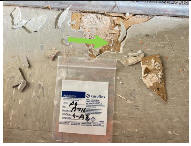
Photograph 14 (20.06.024): Representative photo of the brown-coloured base to vinyl tiles on the internal kitchen floor, Sample ID: 4-A3 (NAD).
