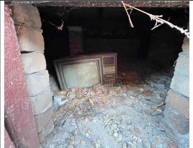
Photograph 22 (20.06.24): Representative photos of basement of building structure located at 56 Yorktown Parade, Maroubra (inaccessible).
