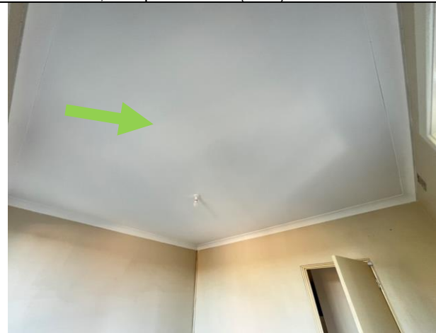
Photograph 16 (20.06.24): Representative photo of white paint system and plasterboard, internal Room 1 ceiling, Sample ID: Lead - Same as 4- LP7 (< 0.01 % w/w) and Asbestos – Same as A1.
