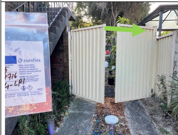
Photograph 3 (20.06.24): Representative photo of yellow paint system, external, northern side gate, Sample ID: 4-LP1 (< 0.01 % w/w)
