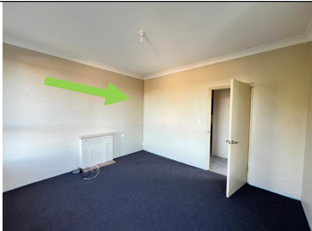
Photograph 17 (20.06.24): Representative photo of yellow paint system, internal room 1 walls on all 4 walls, Sample ID: same as 4- LP 8 (< 0.01 % w/w).
