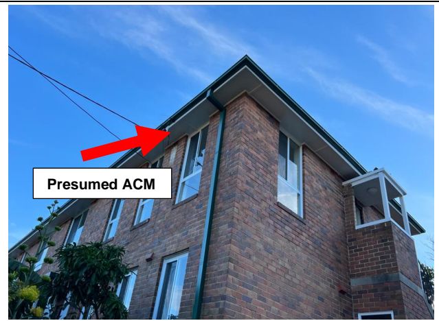
Photograph 2 (20.06.24): Representative photos of White coloured fibre cement sheeting board, External, Roof- Eaves; Sample ID: Visual Only (Presumed ACM)
