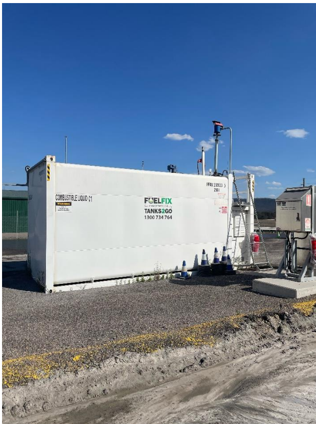
Plate 4 Bunded chemical storage container at LV refuel point
