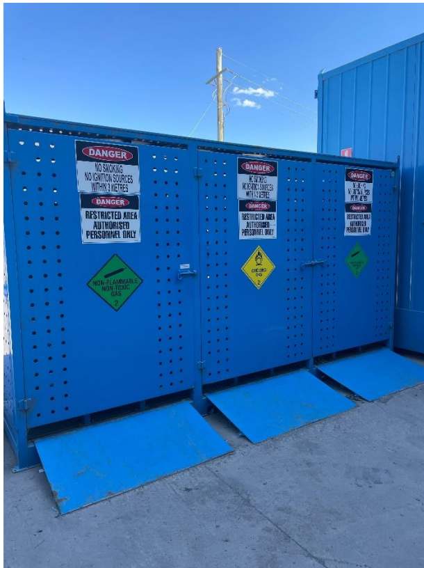
Plate 5 Bunded Chemical Storage
