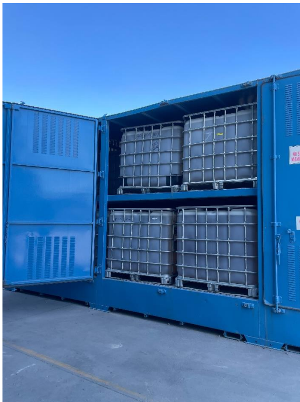
Plate 6 Bunded chemical storage (opened)
