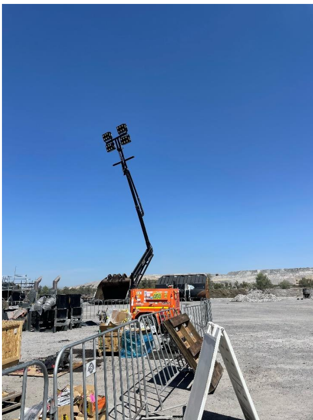
Plate 12 Mobile lighting plant at excavator maintenance pad
