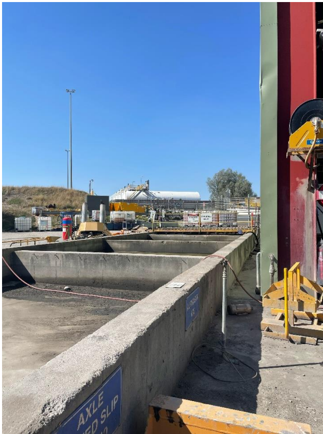
Plate 1 Bunded chemical storage area
