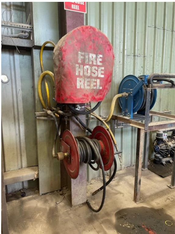
Plate 10 Fire hose available within UWJV workshop
