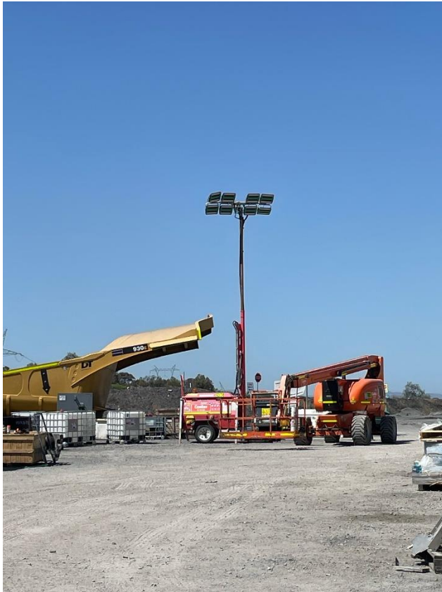
Plate 13 Mobile lighting plant at laydown area
