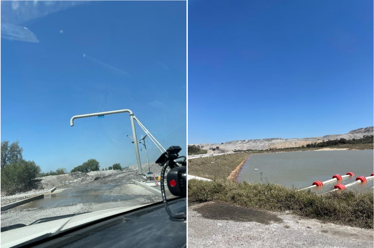
Plate 29 Water Fill and Transfer Points
