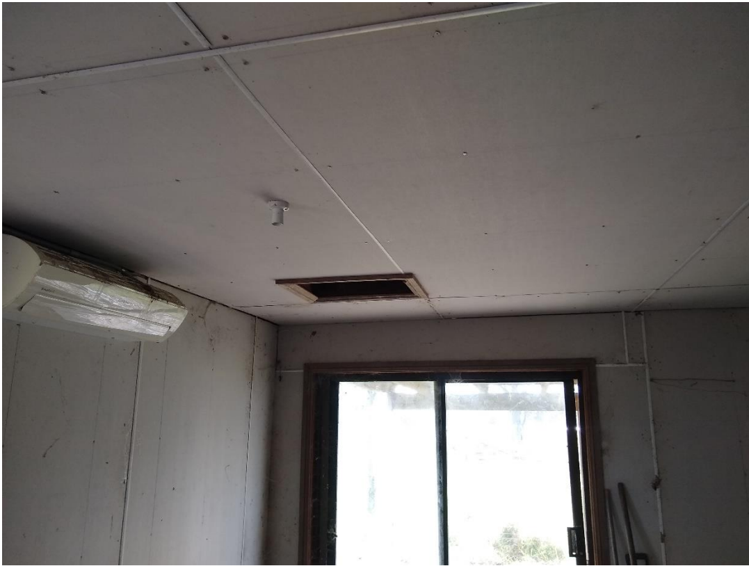
Photo 67: Building GS, ceiling cavity, throughout ceiling cavity, insulation generally, SMF (suspected)
