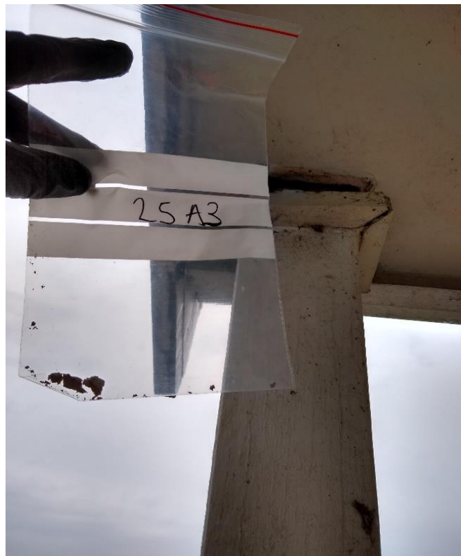
Photo: 16 Building 25, exterior, sheeting from eaves, fibre cement sheeting, sample 25A3, asbestos detected by analysis.
