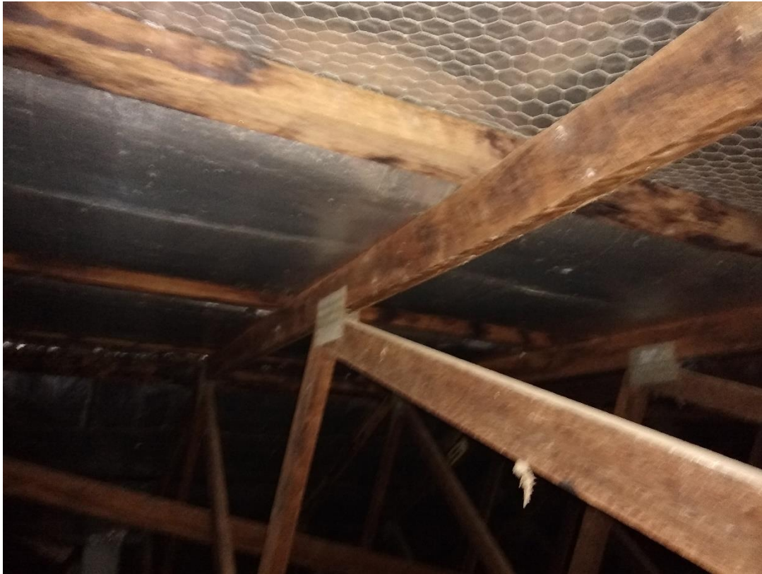
Photo 65: Building 25, ceiling cavity, throughout ceiling cavity, insulation generally, SMF (suspected)
