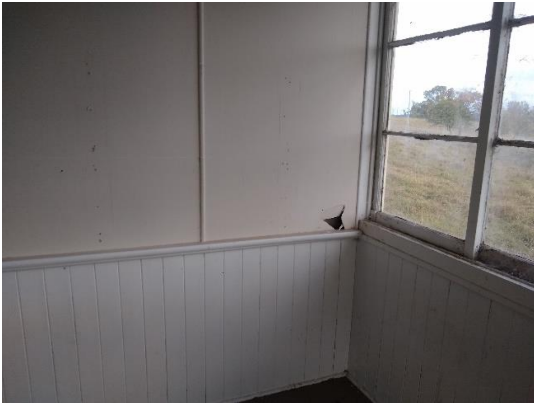
Photo 25: Building HS, interior, sheeting from partition in western portion of house, fibre cement sheeting, sample HSA4, asbestos detected by analysis.
