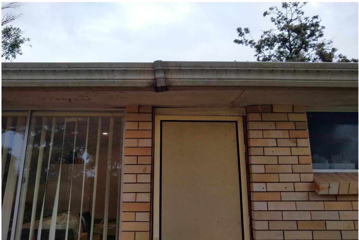
Photo 8: Building 11, exterior, sheeting from eaves, fibre cement sheeting, sample 11A4, asbestos detected by analysis.
