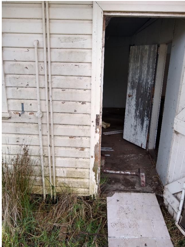
Photo 46: Building GS, exterior, paint off timber door on southern side of garage structure, white paint, sample GSL2, lead paint(s) identified
