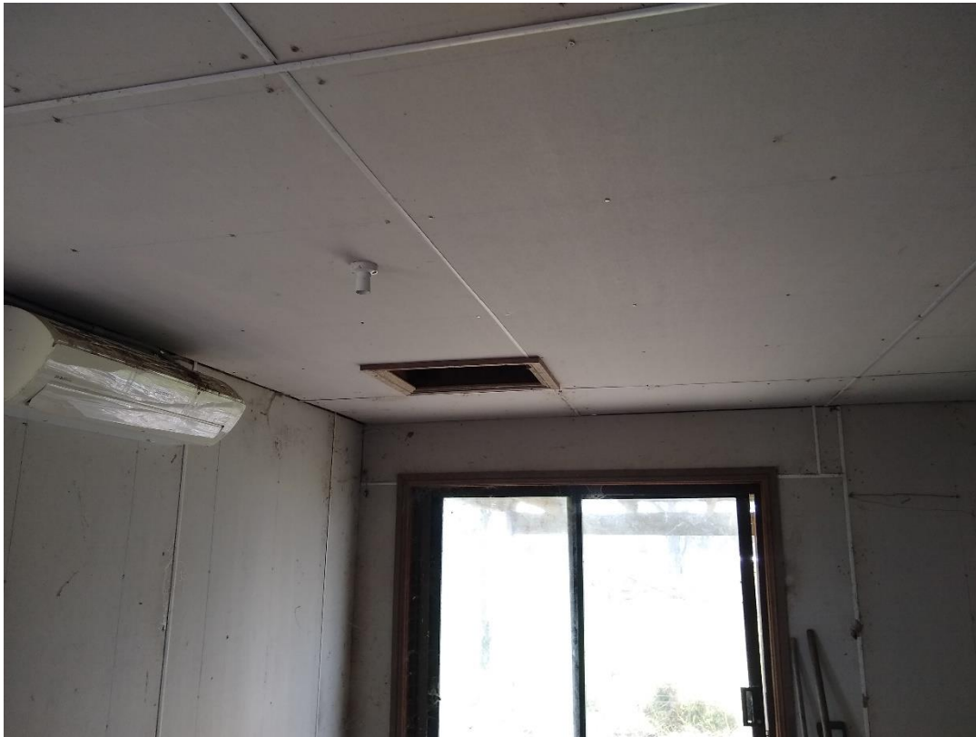
Photo 57: Building GS, manhole on garage ceiling, throughout, settled dust, sample GSD1, elevated lead concentration ( \geq 0.5 mg/m 2 )
