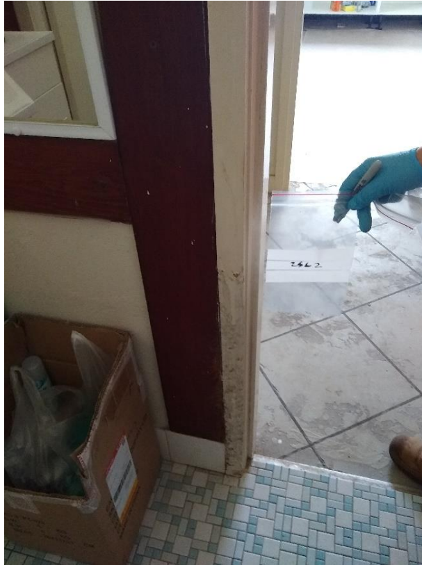
Photo 37: Building 25, interior, paint off timber door frame in southern portion of house, white paint, sample 25L2, lead paint(s) identified
