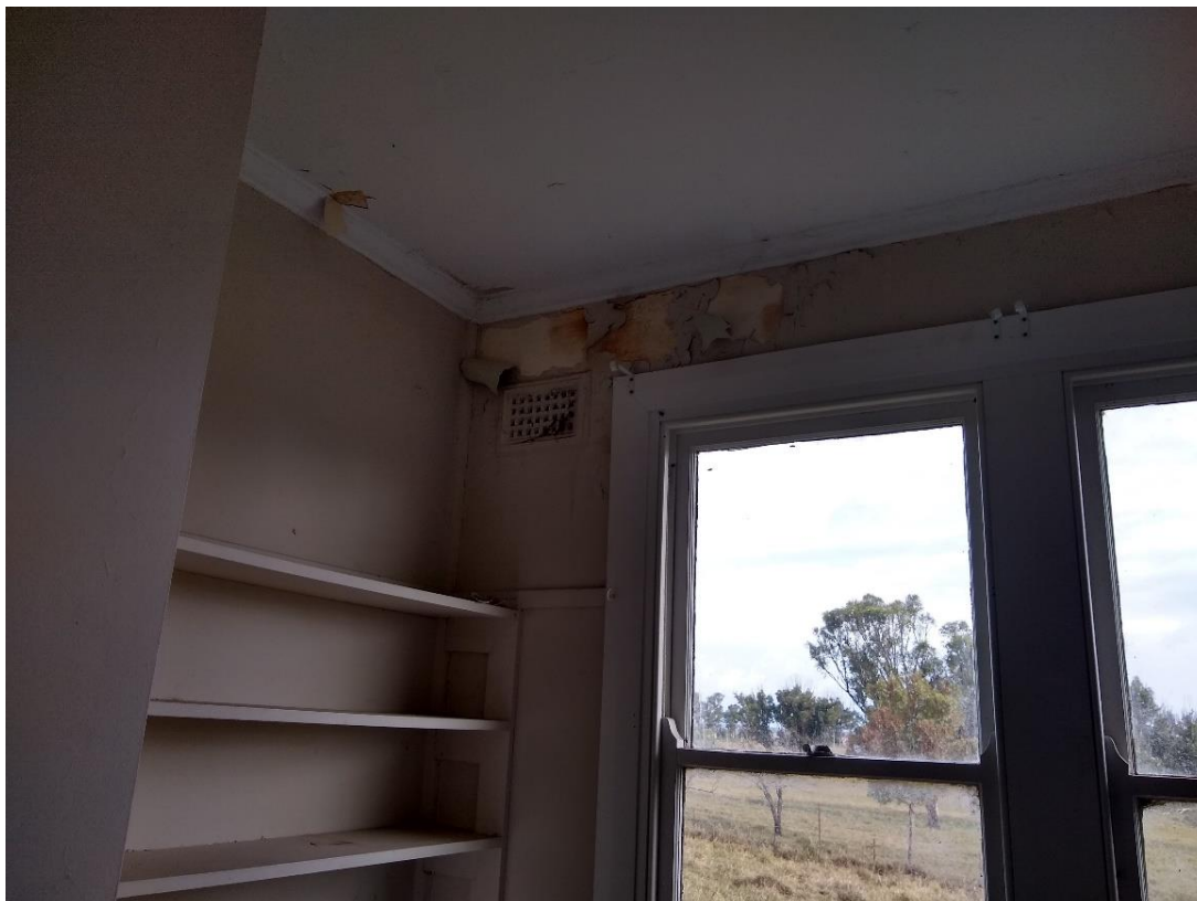
Photo 44: Building HS, interior, paint off wall on southern side of house, white paint, sample HSL4, lead paint(s) identified
