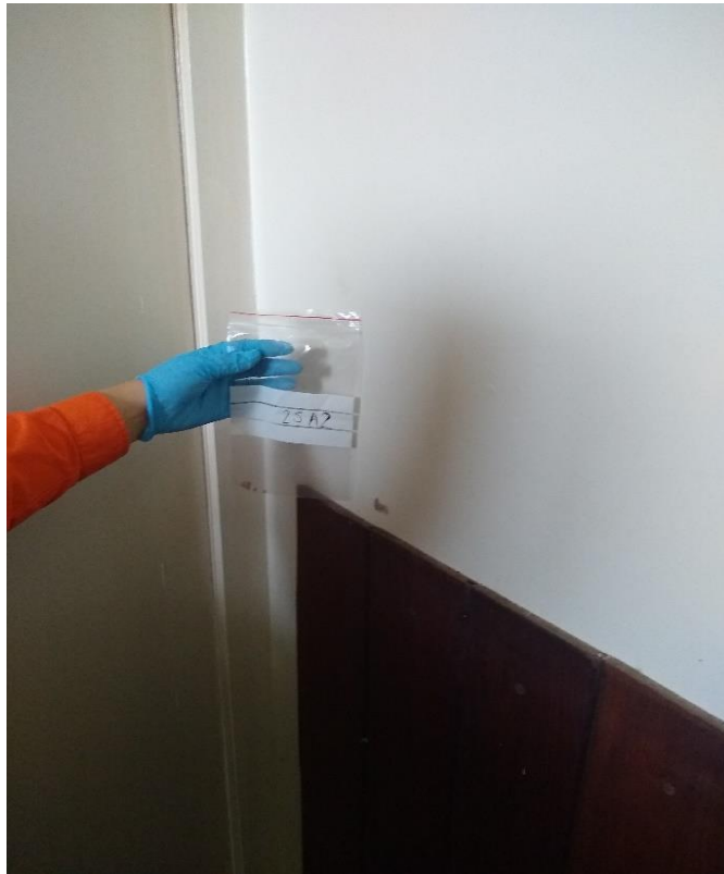
Photo 15: Building 25, interior, wall sheeting in southern portion of house, fibre cement sheeting, sample 25A2, asbestos detected by analysis.
