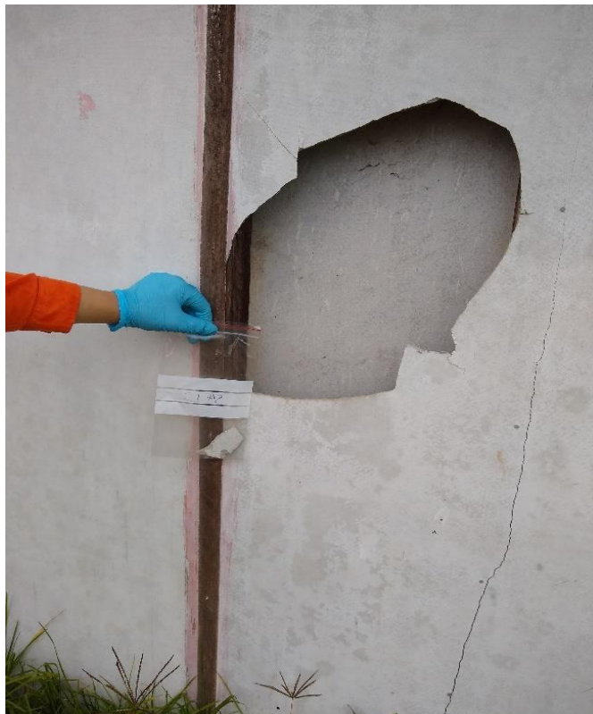
Photo 10: Building 21, exterior, wall sheeting on side shed, fibre cement sheeting, sample 21A2, asbestos detected by analysis.
