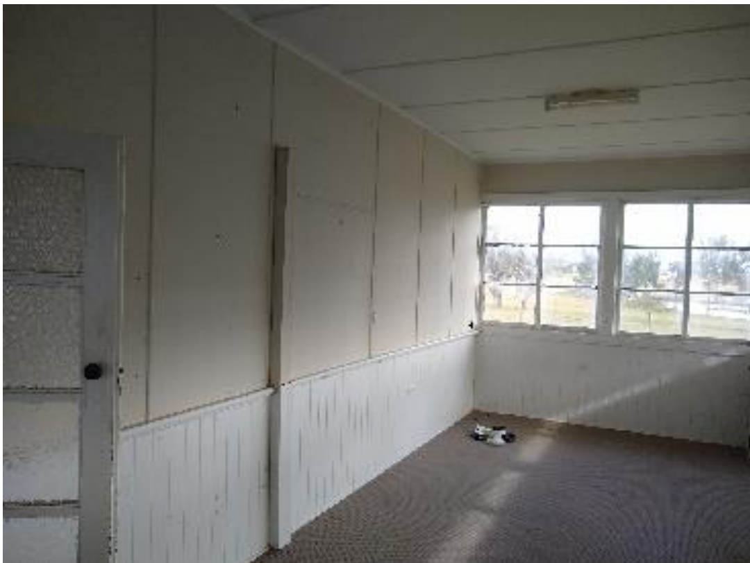
Photo 62: Building HS, interior , western portion of house, fluorescent light fittings, internal components, nil PCB (suspected)
