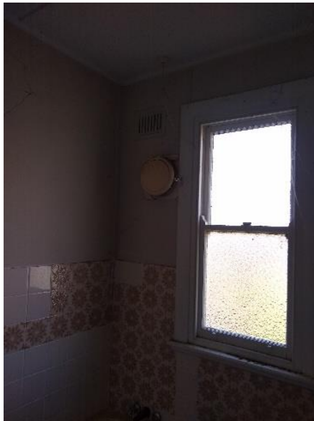
Photo 56: Building HS, ventilation grate in bathroom, throughout, settled dust, sample HSD2, elevated lead concentration ( \geq 0.5 mg/m 2 )
