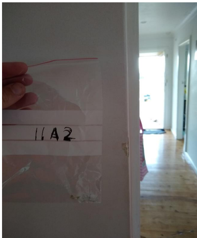
Photo 6: Building 11, interior, wall sheeting within eastern corridor of house, fibre cement sheeting, sample 11A2, asbestos detected by analysis.
