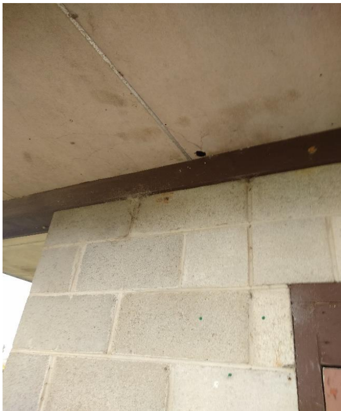
Photo 17: Building 34, exterior, sheeting from eaves, fibre cement sheeting, sample 34A1, asbestos detected by analysis.
