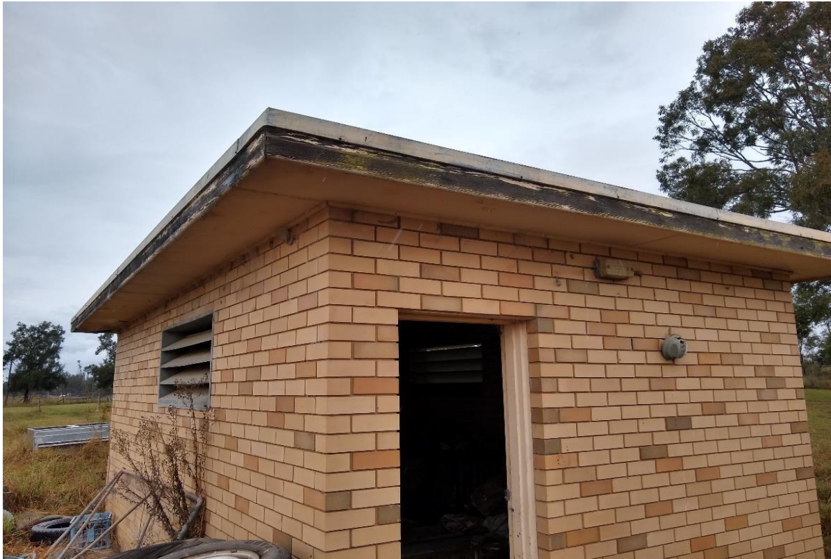
Photo 21: Building 23a, exterior, sheeting from eaves, fibre cement sheeting, N/A, suspected asbestos.
