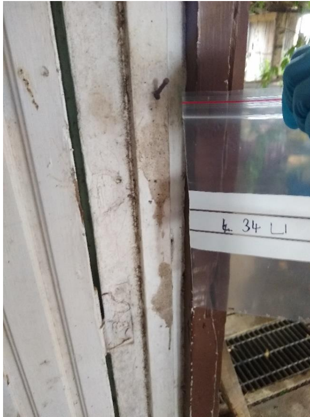
Photo 39: Building 34, interior, paint off timber door frame on eastern side of structure, brown paint, sample 34L1, lead paint(s) identified
