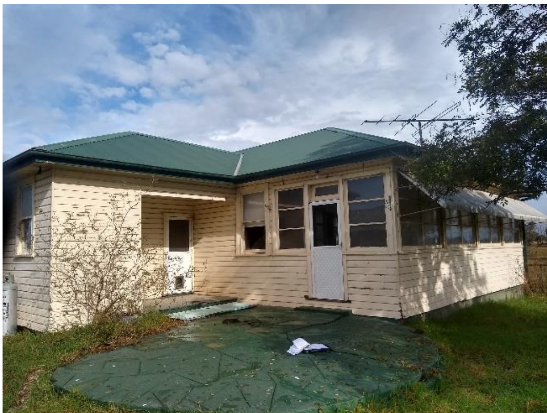
Photo 41: Building HS, exterior, paint off timber on northern side of house, beige paint, sample HSL1, lead paint(s) identified
