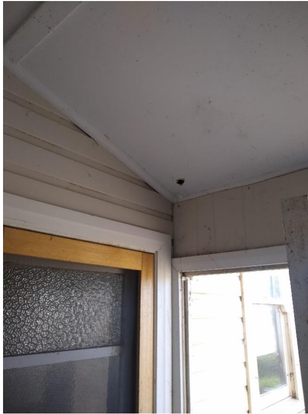
Photo 23: Building HS, interior, sheeting from ceiling near central northern entrance to house, fibre cement sheeting, sample HSA2, asbestos detected by analysis.
