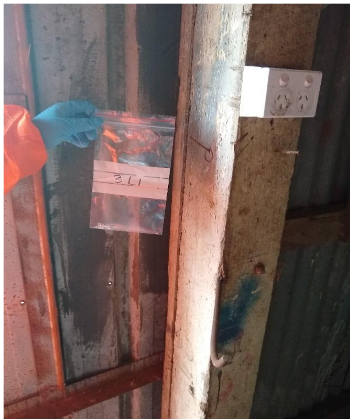
Photo 28: Building 3, interior, paint off timber post in western portion of shed structure, light red paint, sample 3L1, lead paint(s) identified
