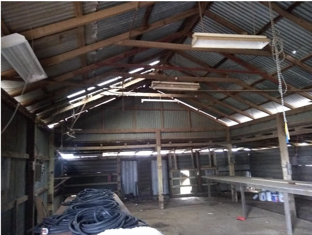
Photo 59: Building 3, interior , throughout, fluorescent light fittings, internal components, inaccessible
