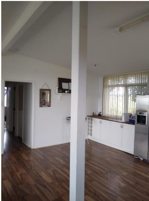
Photo 61: Building 24, interior , central portion of house, fluorescent light fittings, internal components, nil PCB (suspected)
