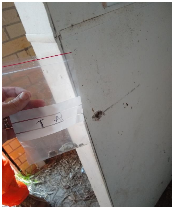
Photo 20: Toilet (T), interior, sheeting from wall, fibre cement sheeting, sample TA1, no asbestos detected by analysis.
