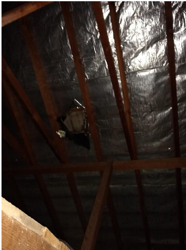
Photo 63: Building 11, ceiling cavity, throughout ceiling cavity, insulation generally, SMF (suspected)
