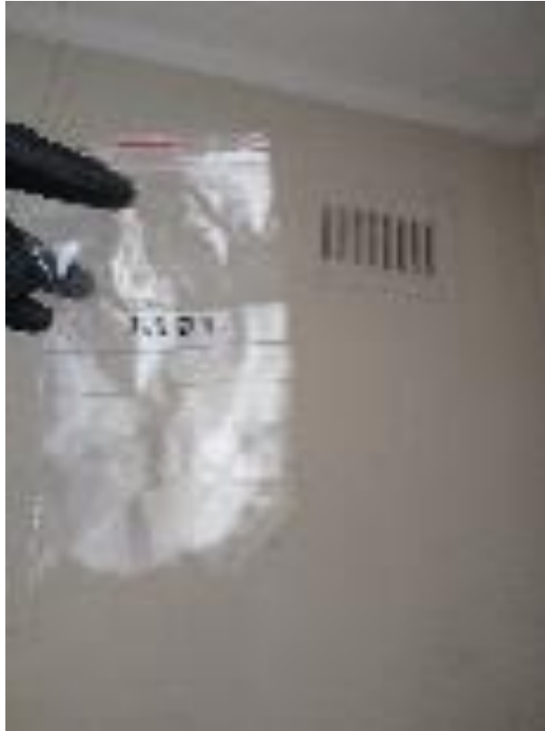
Photo 55: Building HS, ventilation grate in kitchen, throughout, settled dust, sample HSD1, elevated lead concentration ( \geq 0.5 mg/m 2 )
