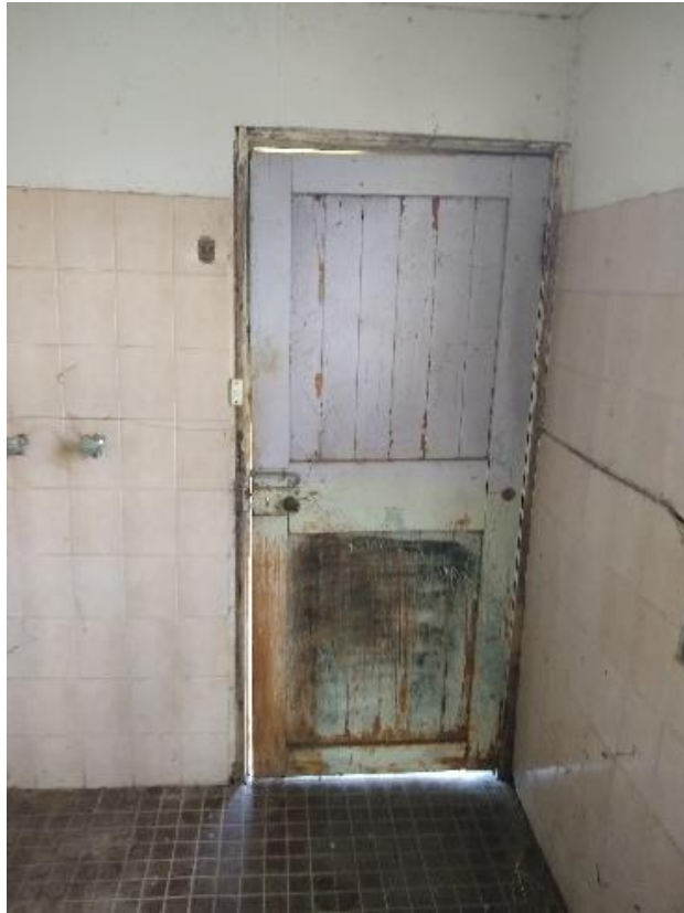
Photo 45: Building GS, interior, paint off timber door on eastern side of garage structure, white paint, sample GSL1, lead paint(s) identified
