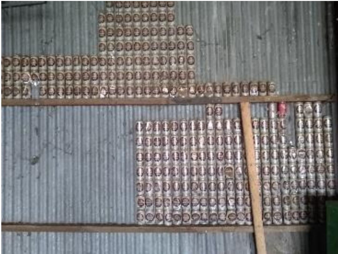
Photo 47: Building 2, timber frame on eastern side of shed, throughout, settled dust, sample 2D1, elevated lead concentration ( \geq 0.5 mg/m 2 )
