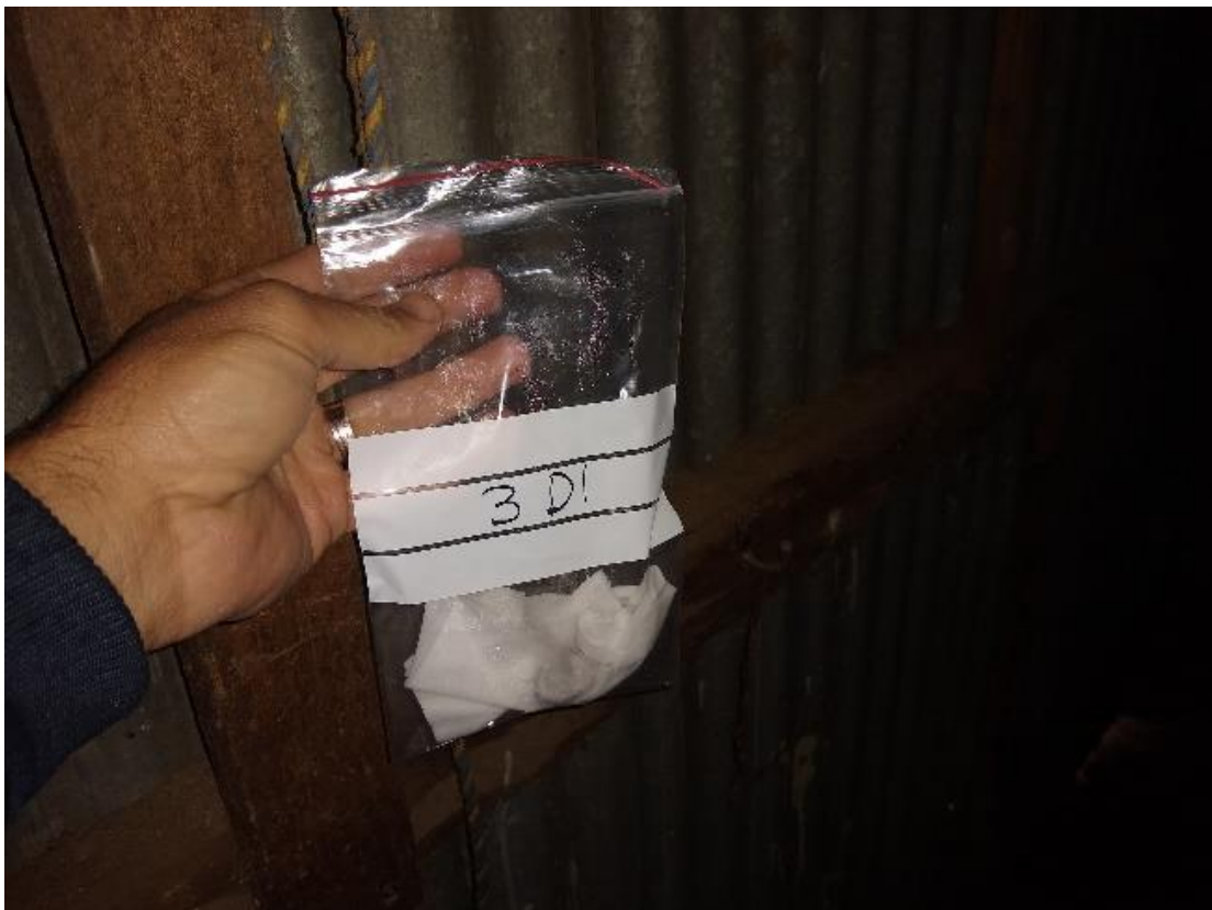
Photo 48: Building 3, timber frame on western side of shed, throughout, settled dust, sample 3D1, elevated lead concentration ( \geq 0.5 mg/m 2 )
