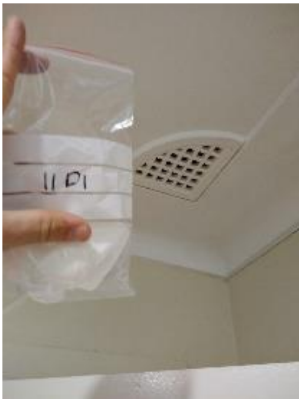
Photo 49: Building 11, ventilation grate in front bedroom, throughout, settled dust, sample 11D1, lead concentration <0.5 mg/m2
