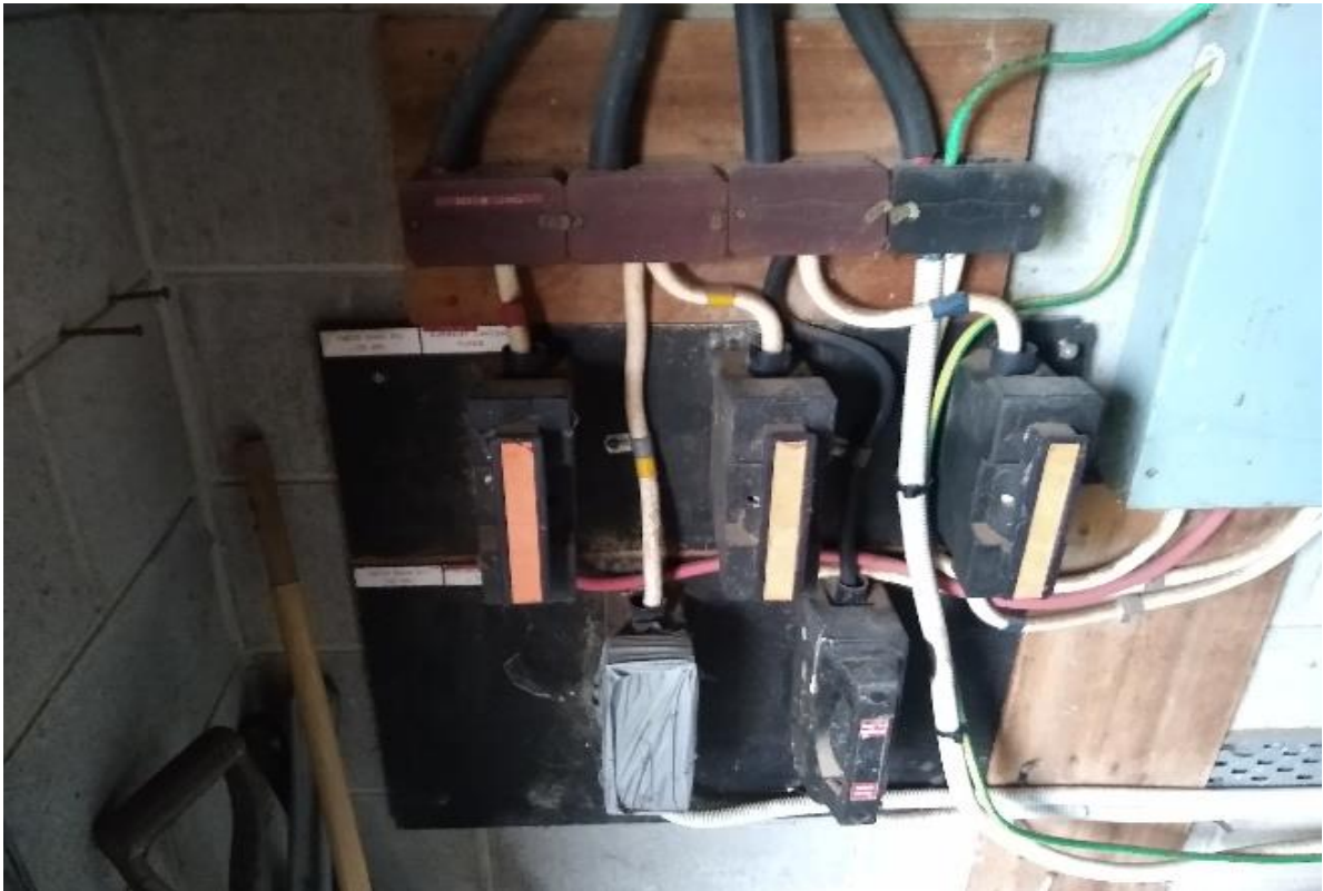
Photo 19: Building 34, interior, backing board from electrical box, black bituminous material, sample 34A3, asbestos detected by analysis.
