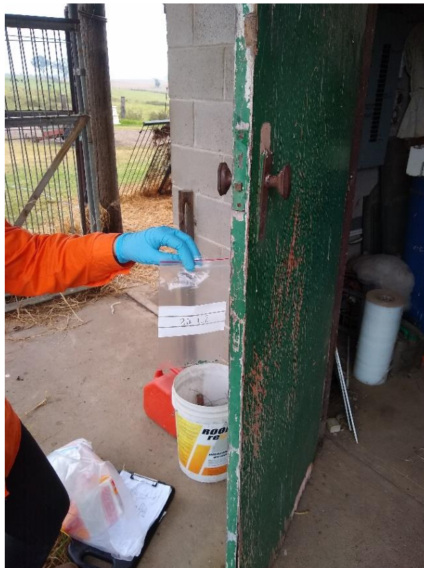
Photo 40: Building 34, exterior, paint off timber door, green paint, 34L2, lead paint(s) identified
