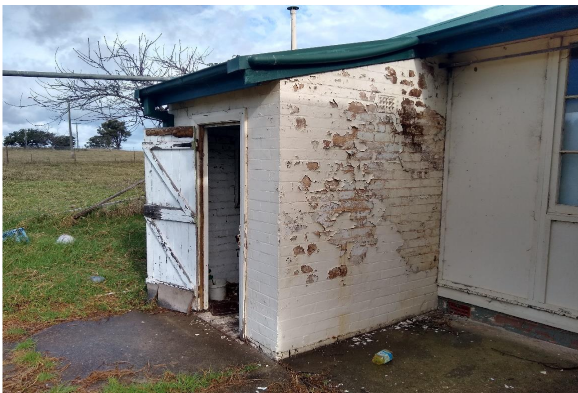
Photo 42: Building HS, exterior, paint off brickwork on exterior toilet, beige paint, sample HSL2, lead paint(s) identified
