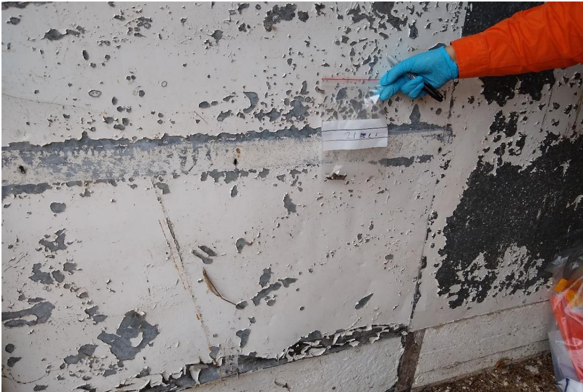
Photo 68: Building 21, interior, paint off wall within southern portion of shed, white paint, sample 21L1, lead paint(s) identified
