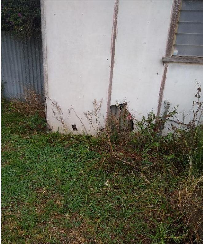
Photo 9: Building 21, exterior, wall sheeting on side shed, fibre cement sheeting, sample 21A1, asbestos detected by analysis.
