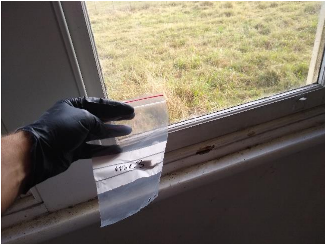
Photo 43: Building HS, interior, paint off timber window frame on southern side of house, white paint, sample HSL3, lead paint(s) identified
