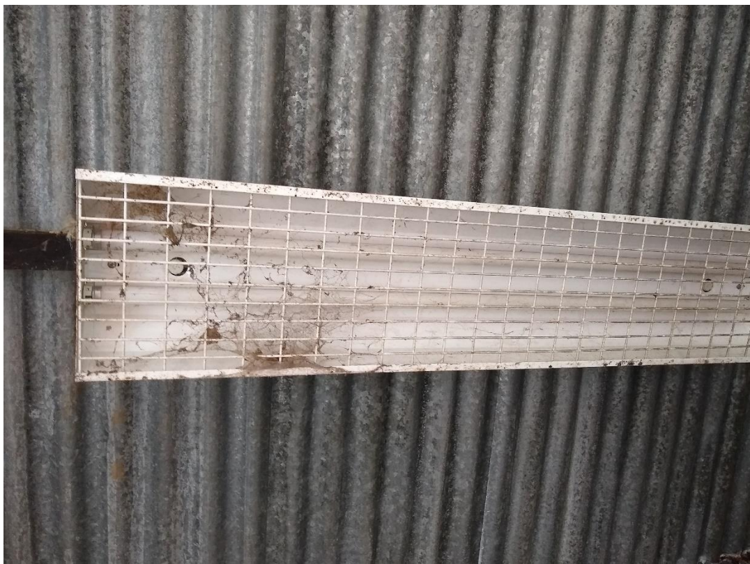
Photo 58: Building 2, interior , eastern portion of shed structure, fluorescent light fittings, internal components, nil PCB (suspected)
