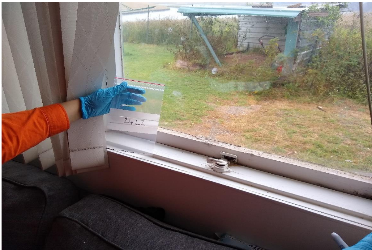
Photo 34: Building 24, interior, paint off timber window frame in southern bedroom in house, white paint, sample 24L2, no lead paint(s) identified
