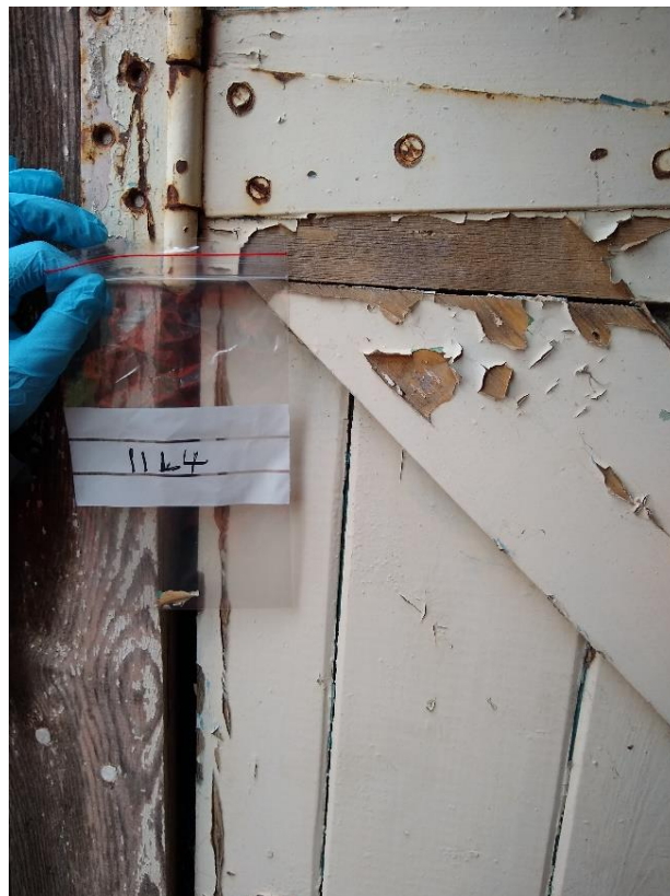
Photo 32: Building 11, exterior, paint off timber exterior door on southern side of dwelling, white paint, sample 11L4, lead paint(s) identified
