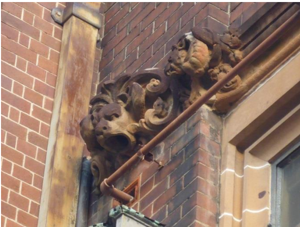
PICTURE 17 – DETAIL OF ONE OF THE GARGOYLES (MISSING DP) AND SERVICES (DRENCHERS)
