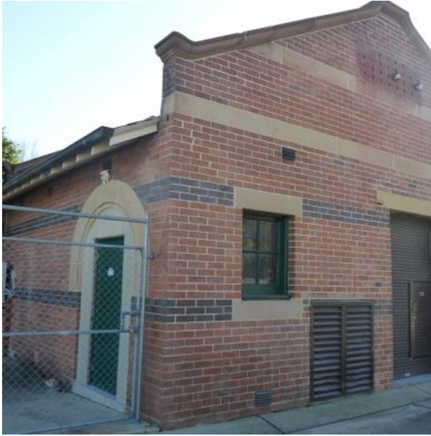
PICTURE 9 – VIEW TOWARDS THE SOUTH WEST CORNER OF THE SUBSTATION.
