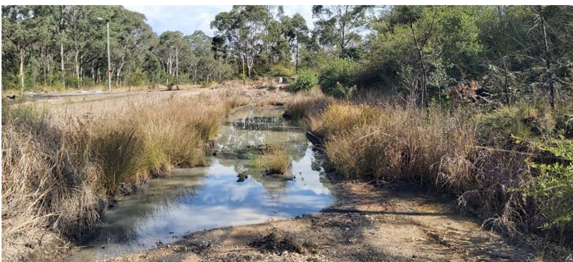
Photograph 3 Subsided mine entry adjacent to rail line (Village 3 Area)
