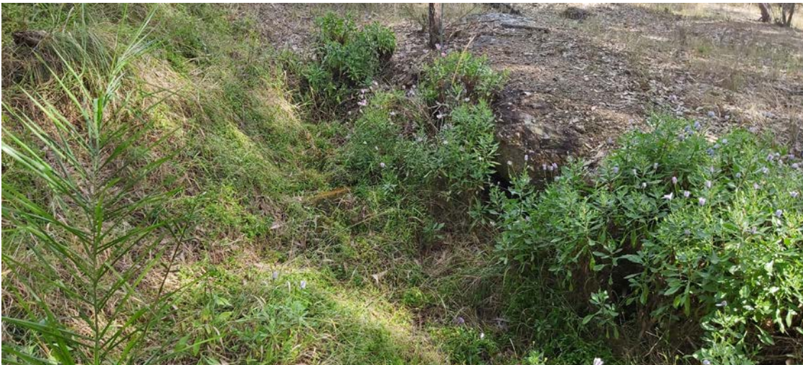
Photograph 5 Apparent subsidence scarp in the Stage 2 North area (Village 3 Area)
