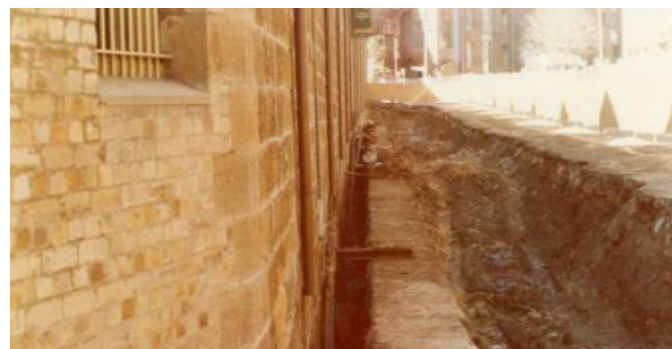
Figure 2.1 Photograph of Hickson Road works from the 1980's showing the non-existent dwarf sandstone walls. (extract from CMP p. 89, Figure CCM 172 (SHFA))
