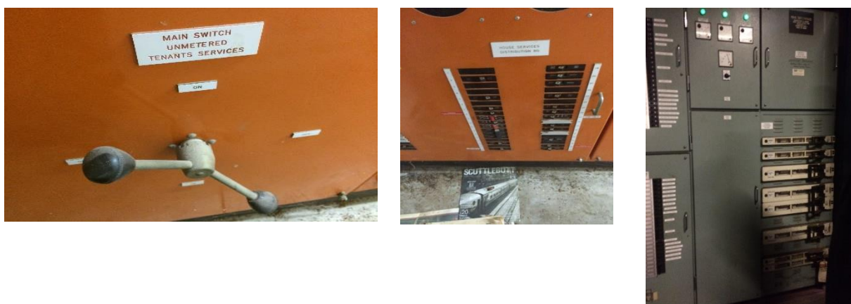
Figure 3.4 – Existing main switchboards and distribution boards
