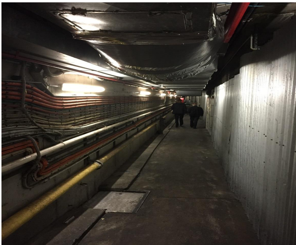
Figure 3.2 – Existing gas main within service corridor
