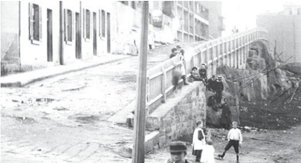
PICTURE 25 – C1901 SHOWING THE CUTTING BACK OF THE ROCK FACE ON HARRINGTON STREET AND PARTIAL CONSTRUCTION OF THE STONE FACING OF THE WALL (SOURCE : CUMBERLAND PLACE CMP SHFA 2008).
