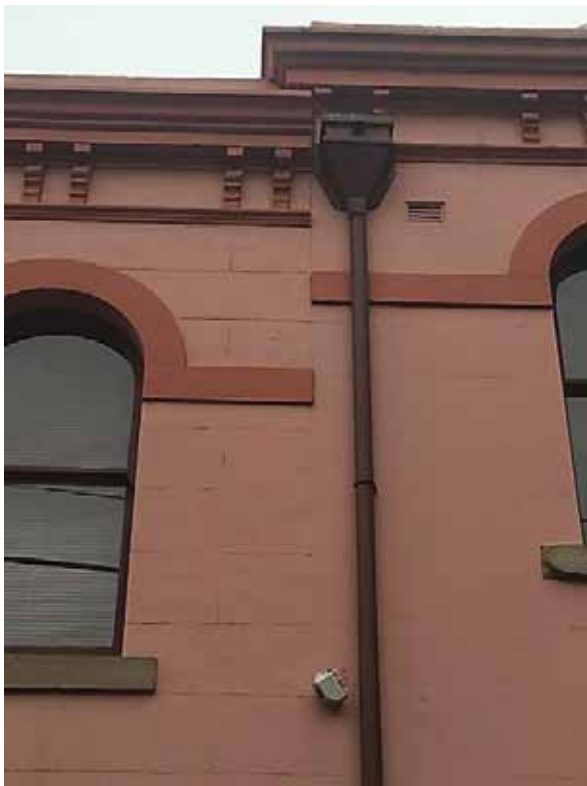
PICTURE 19 – DETAIL FRONT (EAST) FAÇADE SHOWING PAINTED RENDERED MASONRY AND CORNICE ETC. (NOVEMBER 2015)
