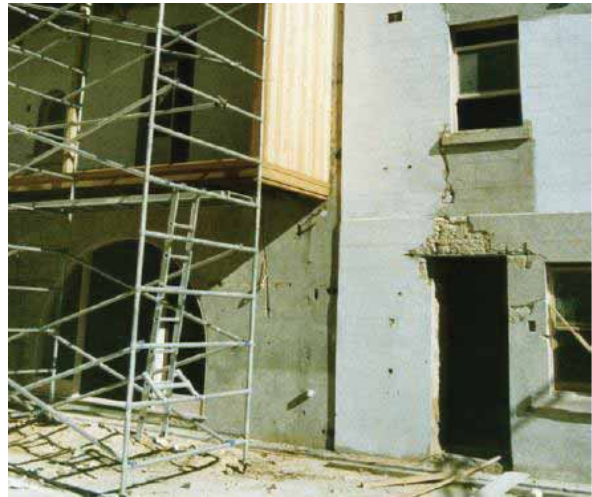
PICTURE 81 – REAR FAÇADE IMMEDIATELY SHOWING RESTORATION, 1991. NOTE MUCH OF THE EXTERNAL RENDER APPEARS TO HAVE BEEN REPLACED (SOURCE: BAKERS TERRACE CMP, 2007)
