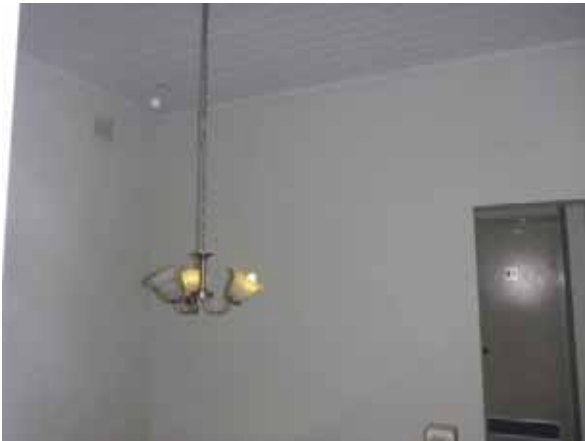
PICTURE 59 – SPACE G5 FACING NORTH EAST (VIEW FROM LEVEL ABOVE). NOTE MODERN LIGHTING AND TIMBER BEADED CEILING. (NOVEMBER 2015)
