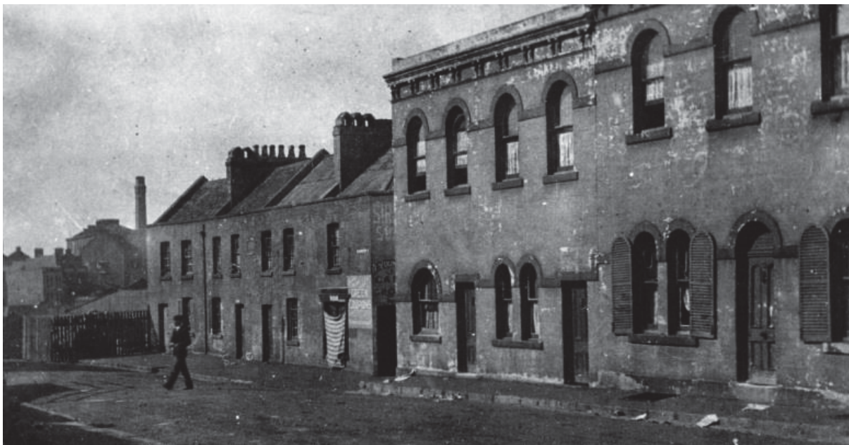
FIGURE 27 – GLOUCESTER STREET SHOWING BAKERS TERRACE. THEY ARE NOTED TO BE VERY DILAPIDATED AND WITH SHUTTERS ON THE LOWER LEVEL SOUTHERN TERRACES.
