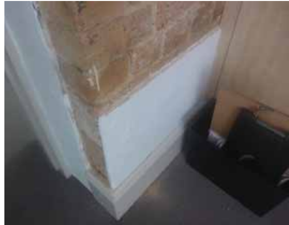
PICTURE 40 – VIEW OF REMNANT PLASTERWORK ON WESTERN ROOM OF SPACE 52 (NOVEMBER 2015)
