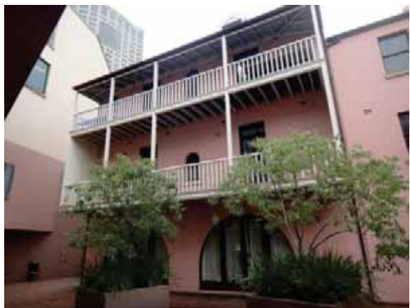
PICTURE 26 – DETAIL OF REAR BALCONY RECONSTRUCTED IN THE LATE 1980S WORKS. (NOVEMBER 2015)
