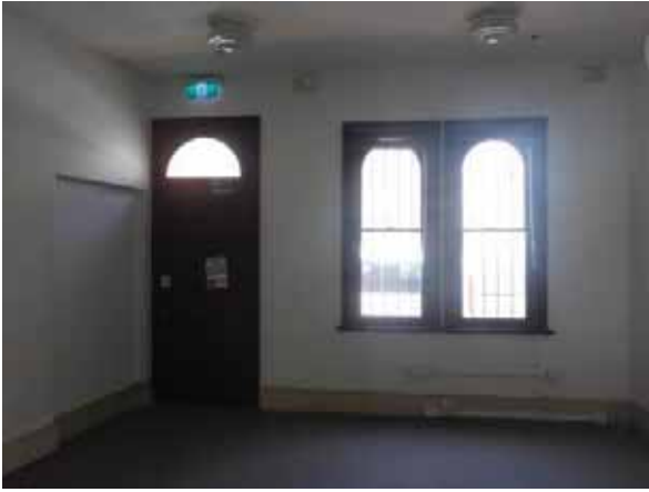
PICTURE 55 – SPACE G3 FACING WEST. NOTE INFILLED SECTION OF SOUTHERN WALL. (NOVEMBER 2015)
