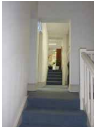
PICTURE 60 – SPACE G5 FACING SOUTH. VIEW AT TOP OF STAIRS LOOKING TOWARDS FIRST FLOOR LEVEL. (NOVEMBER 2015)
