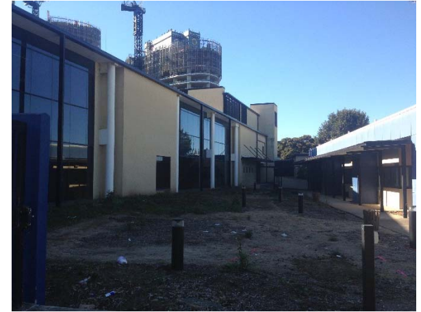
Photograph 3: Southern side of Building one with suspected asbestos eaves and third level containing the air-conditioning units.
