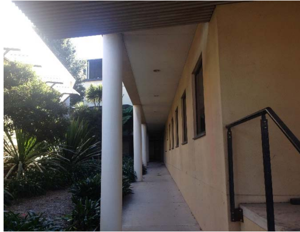
Photograph 14: Western side of Building one with suspected asbestos sheeting
