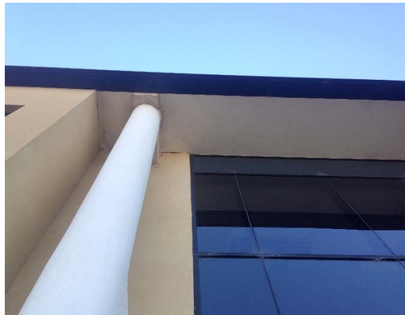
Photograph 5: Suspected asbestos eaves on the southern side of Building one
