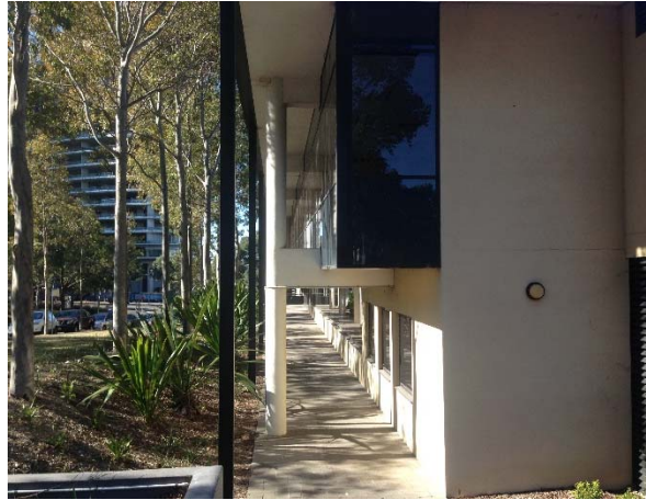
Photograph 2: Northern side of Building one with suspected asbestos eaves
