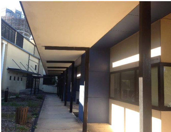
Photograph 10: Suspected asbestos sheeting on the northern side of Building two
