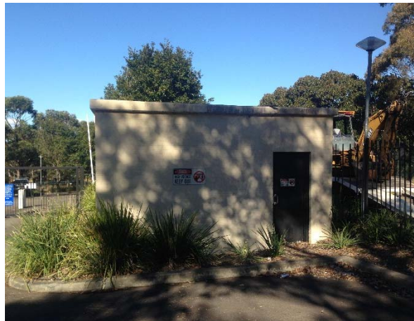
Photograph 11: Northern side of Building three, housing the transformer for the site
