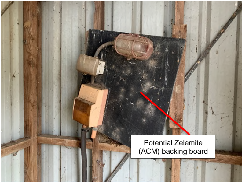
Print 76 Pump house 2 Switchboard on the inside wall.
