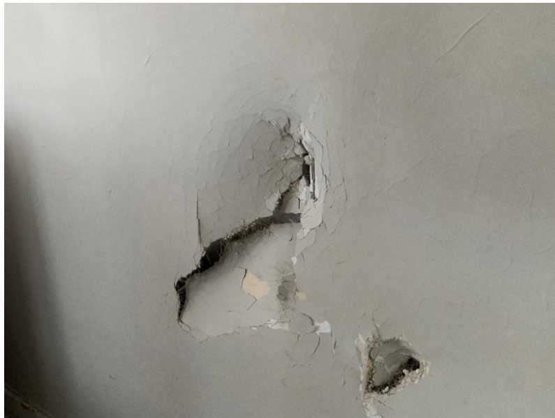
Print 13 Unoccupied house Damaged internal wall in bedroom showing plasterboard composition.
