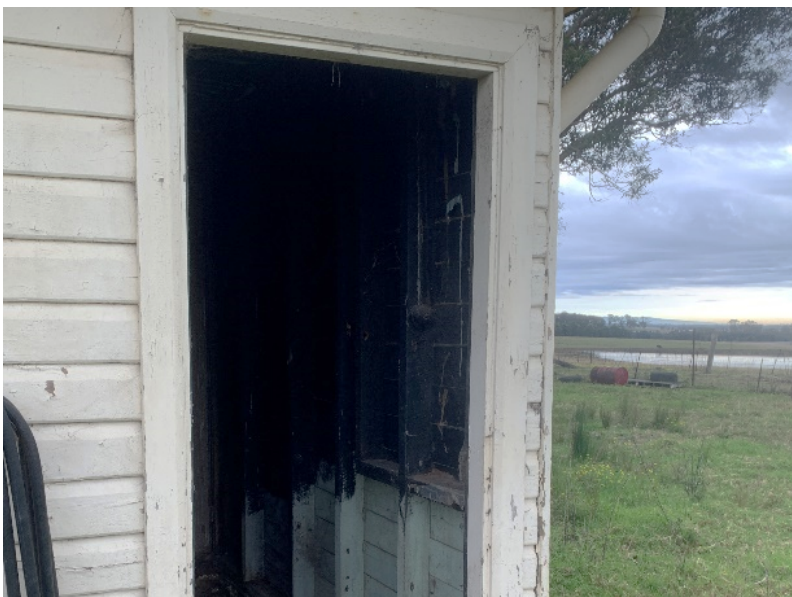
Print 21 Auxiliary building View of the eastern entry to the auxiliary building showing external timber cladding fixed directly to studs.
