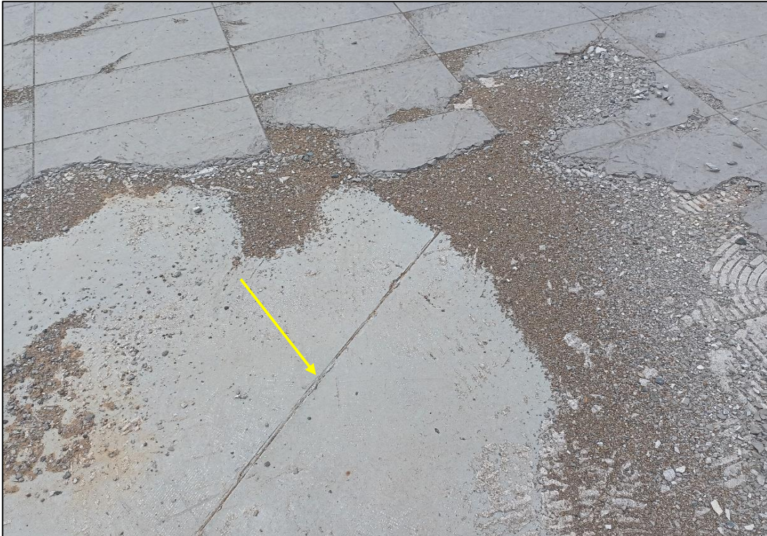
Photo 3: Concrete joints, north-eastern area, jointing, grey mastic, asbestos detected by analysis.
