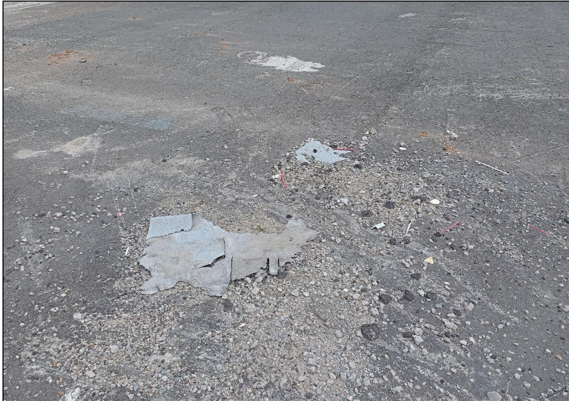
Photo 5: Floor Linoleum, building footprint / north-eastern area, surface, linoleum 2, no asbestos detected by analysis.
