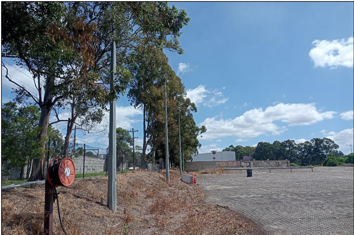
Photo 6: Southern street lights, along northern boundary fence, internal components (e.g. capacitors, ballasts) PCB (suspected).
