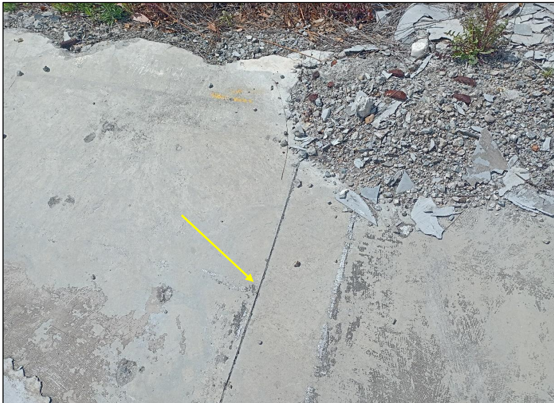
Photo 2: Concrete joints, northern area, jointing, black mastic, asbestos detected by analysis.
