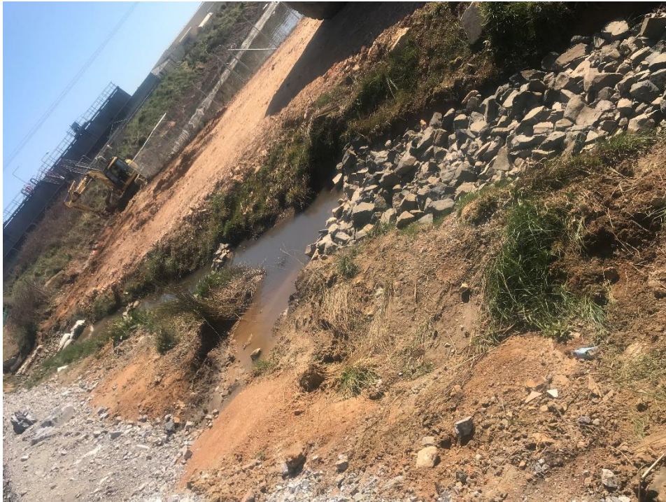
Image 1: Swale drain lined with scour rock
