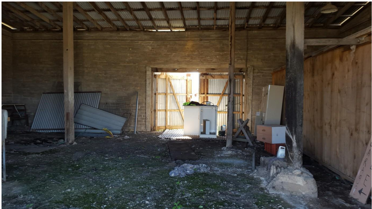
Plate 3.13 Interior of control room showing wooden beams for piles and roof, concrete foundations and dirt floor (20151006_144957).
