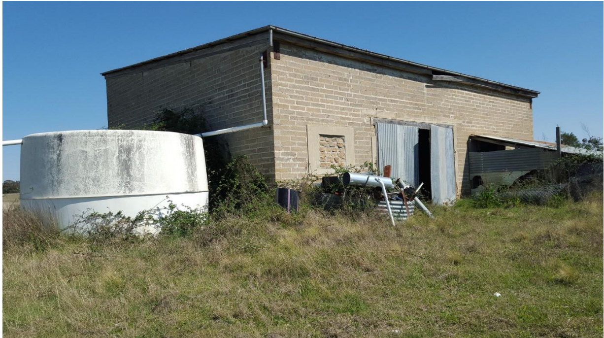
Plate 3.12 Rear of the control room showing corrugated iron engine housing, doors, bricked in openings and a water tank (20151006_145129).
