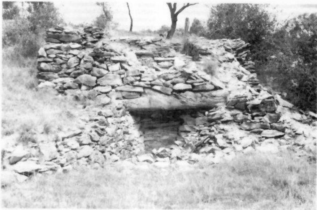
Moses Morley's 1870s kiln on Stringybark Hill south of Queanbeyan. The massive tree trunk supporting the upper part of the kiln's front wall probably helped to stabilise it during the burning process. The front walls of kilns tended to bulge outward with the intense heat. (Photograph by author).
