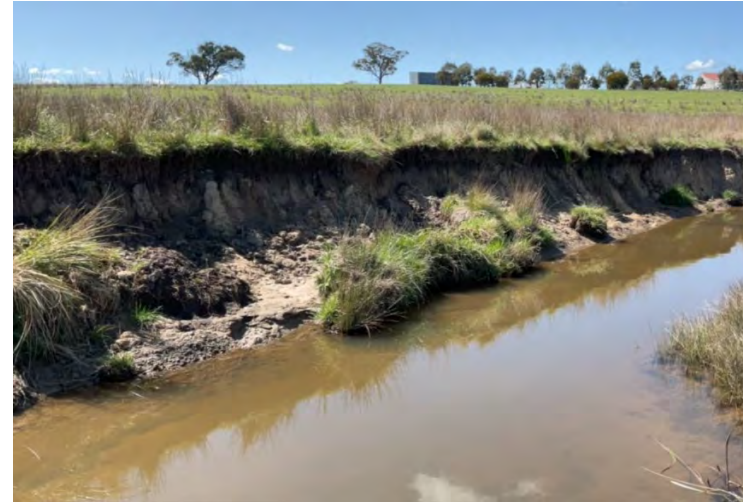
Plate 2 Photo of Duval Creek with bank erosion, facing south, September 2024
