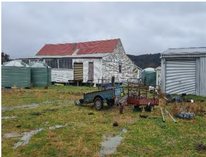
Photo 7 The wool shed is located in the central portion of Lot 4 DP800611. Several aboveground storage tanks and farm equipment were observed in this area. Some flaking paints were also observed in the woolshed. This area is excluded from the development footprint.
