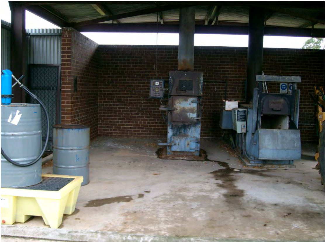
Photograph 8 – Disused incinerator with diesel storage drums in foreground
