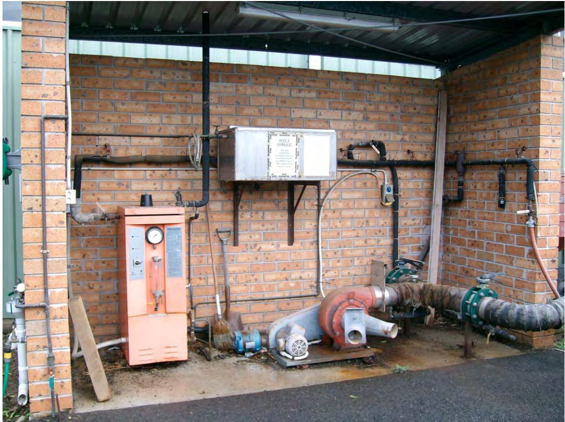
Photograph 3 –Electric sterilising unit with minor staining on the concrete base.
