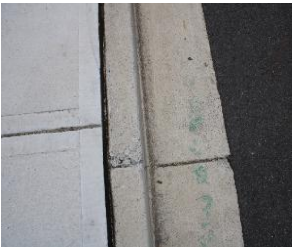
Figure 587 - Crack propagation through kerb and gutter heading North
