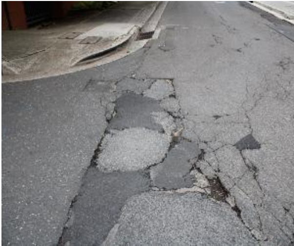
Figure 625 - Crack propagation, patchwork, and loss of materials through road surface heading South
