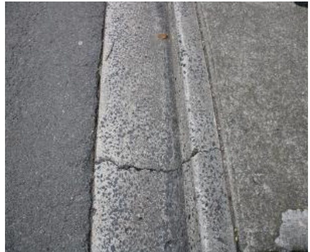
Figure 472 - Crack propagation through kerb and gutter heading North
