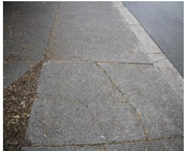
Figure 268 - Crack propagation through footpath pavement heading West
