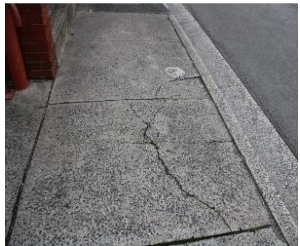
Figure 462 - Crack propagation through footpath pavement heading South
