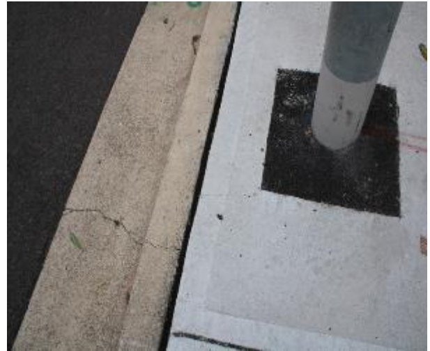
Figure 524 - Crack propagation through footpath pavement heading South
