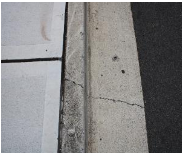
Figure 579 - Crack propagation through kerb and gutter heading North
