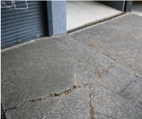
Figure 277 - Crack propagation through footpath pavement heading West
