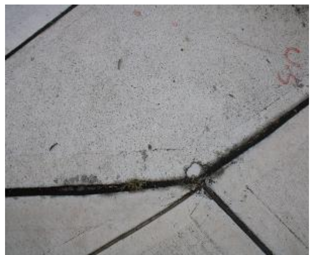
Figure 510 - Crack propagation through footpath pavement heading South
