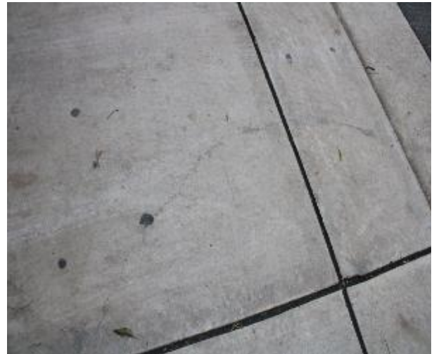
Figure 46 - Crack propagation through driveway pavement heading East
