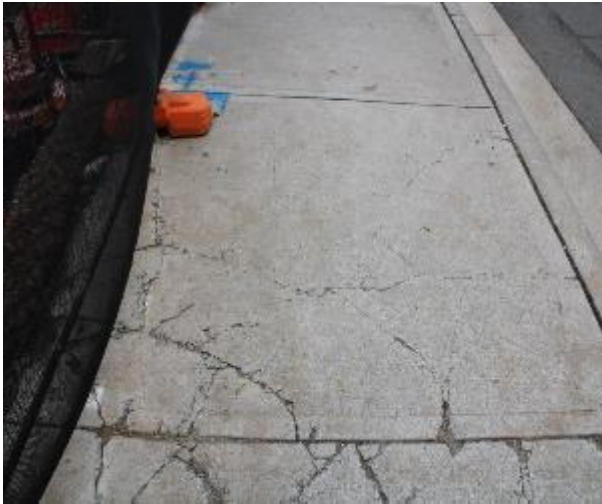
Figure 79 - Crack propagation through footpath pavement heading East
