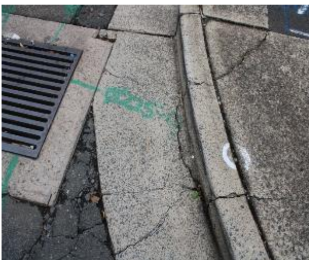
Figure 485 - Crack propagation through kerb and gutter heading North
