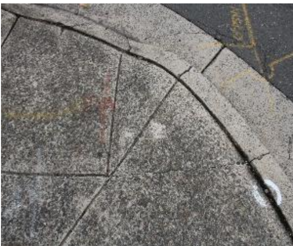
Figure 437 - Crack propagation through footpath pavement heading South
