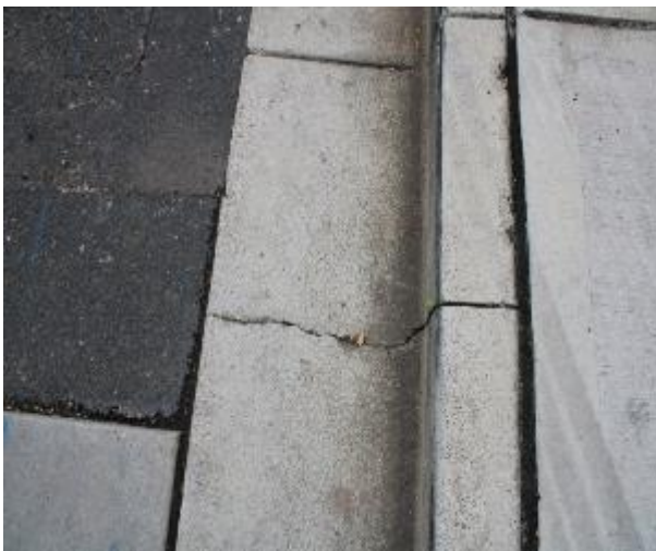
Figure 339 - Crack propagation through kerb and gutter heading East
