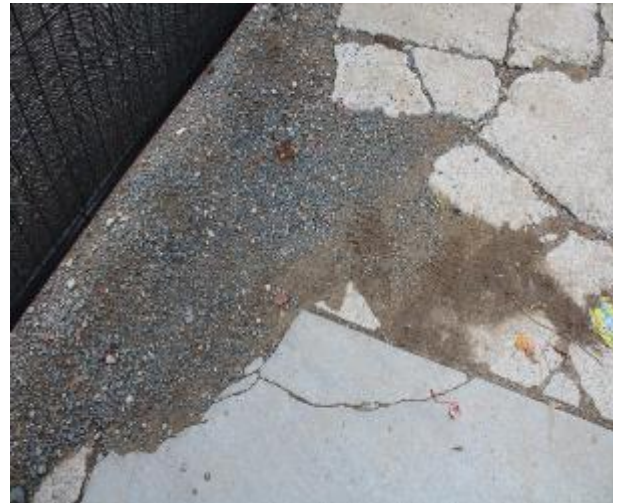
Figure 76 - Crack propagation and loss of materials through footpath pavement heading East
