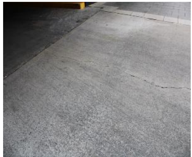
Figure 286 - Crack propagation through footpath pavement heading West
