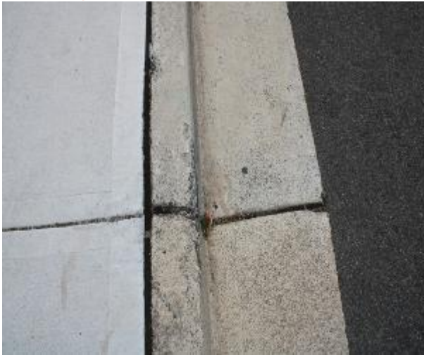
Figure 577 - Crack propagation through kerb and gutter heading North
