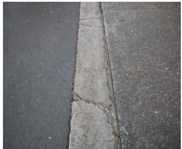
Figure 304 - Crack propagation through kerb and gutter heading East
