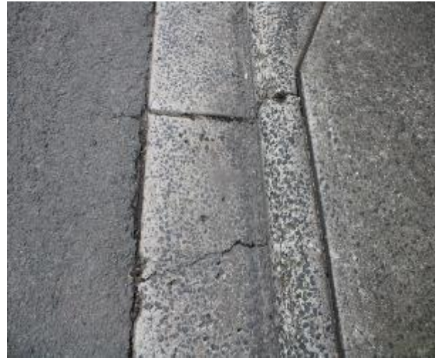
Figure 476 - Crack propagation through kerb and gutter heading North
