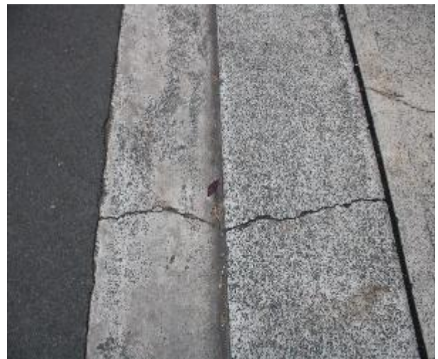
Figure 292 - Crack propagation through driveway layback and gutter heading East
