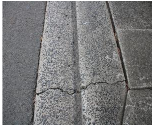
Figure 478 - Crack propagation through driveway layback and gutter heading North
