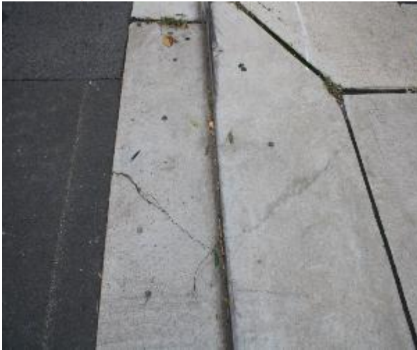
Figure 115 - Crack propagation through driveway layback and gutter heading West
