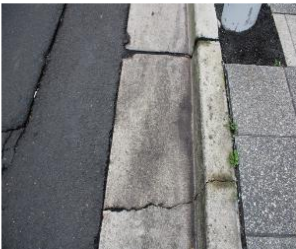
Figure 131 - Crack propagation through kerb and gutter heading West
