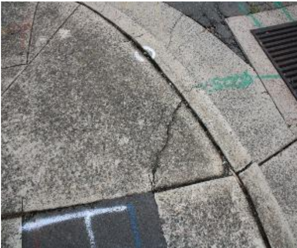
Figure 435 - Crack propagation through footpath pavement heading South
