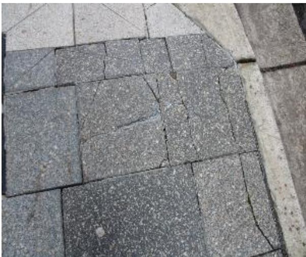
Figure 15 - Crack propagation through footpath pavers heading East
