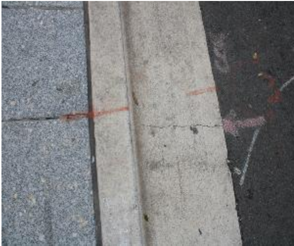
Figure 565 - Crack propagation through kerb and gutter heading North
