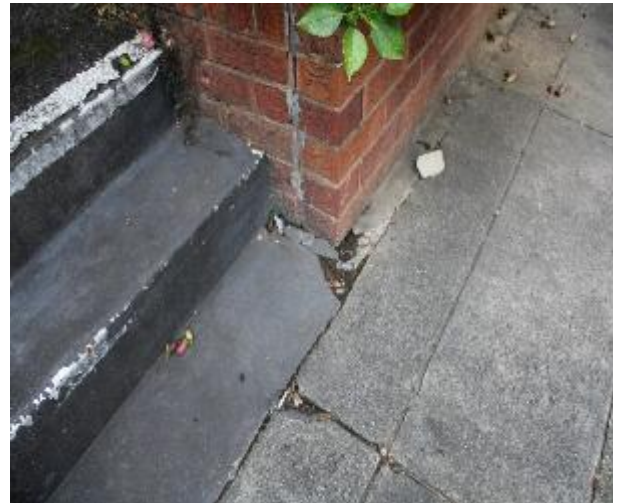
Figure 424 - Loss of material through footpath pavement heading South
