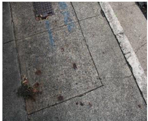
Figure 426 - Crack propagation through footpath pavement heading South
