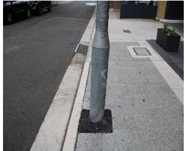
Figure 380 - General condition of street light post Identification No. HR13804
