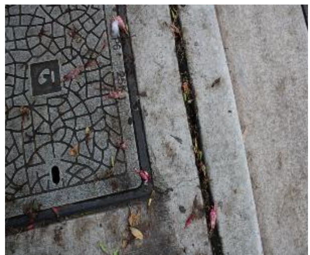
Figure 66 - Crack propagation through footpath pavement heading East
