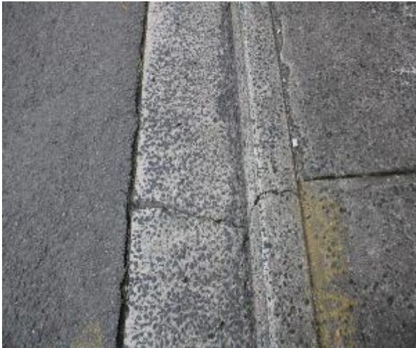
Figure 469 - Crack propagation through kerb and gutter heading North
