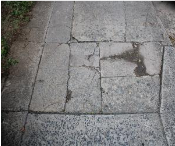
Figure 259 - Crack propagation through footpath pavement heading West
