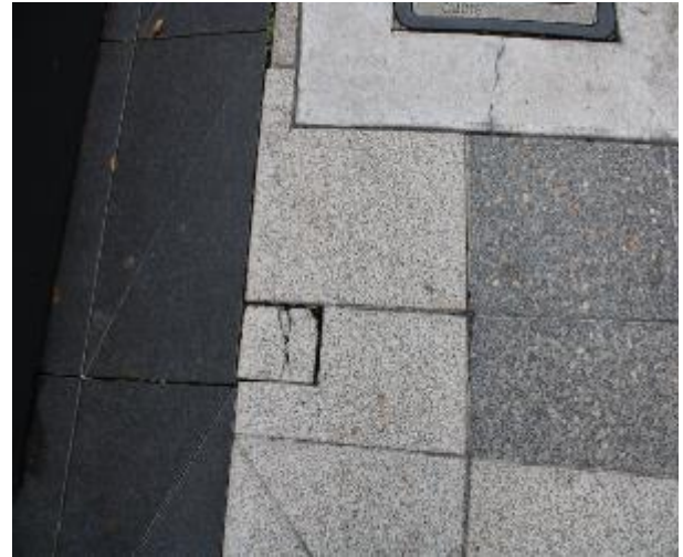
Figure 26 - Crack propagation through footpath pavers heading East
