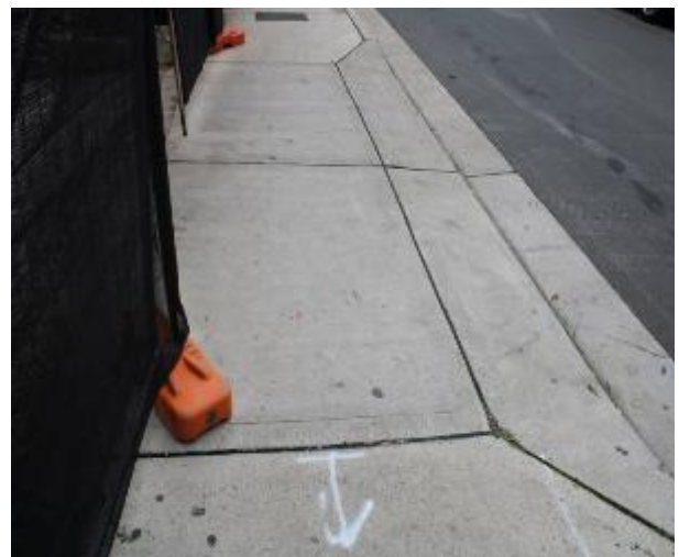
Figure 42 - General condition of driveway pavement heading East
