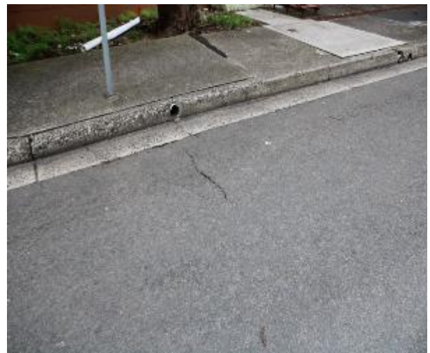
Figure 634 - Crack propagation through road surface heading South
