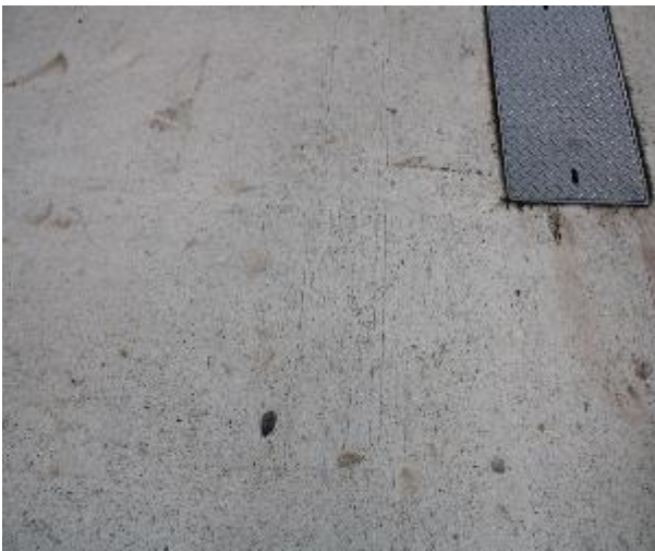
Figure 23 - Crack propagation through driveway pavement heading East
