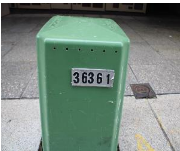
Figure 383 - General condition of electricity box identification No. 36361
