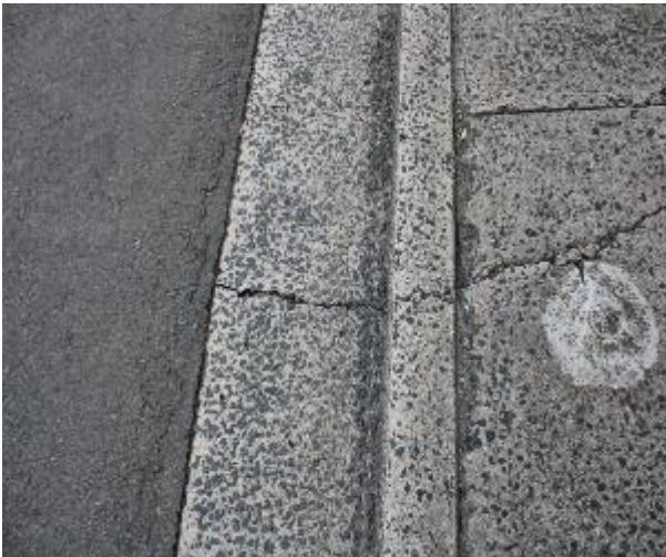
Figure 465 - Crack propagation through kerb and gutter heading North
