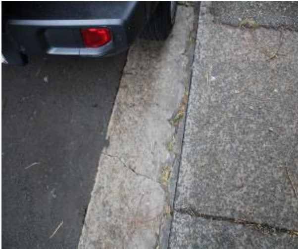
Figure 307 - Crack propagation through kerb and gutter heading East
