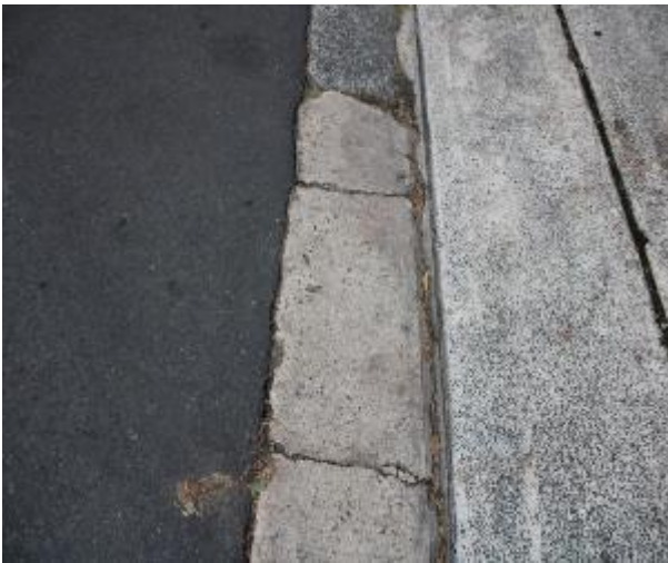
Figure 297 - Crack propagation through driveway layback and gutter heading East
