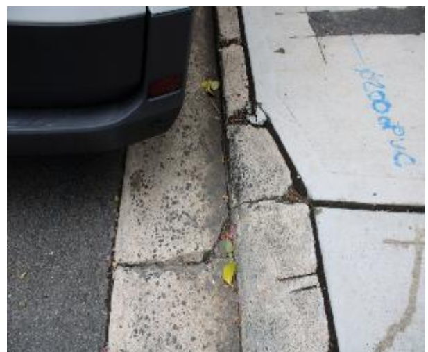
Figure 354 - Crack propagation through driveway layback and gutter heading East
