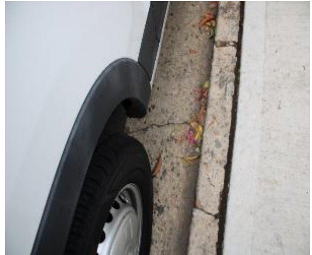
Figure 356 - Crack propagation through kerb and gutter heading East
