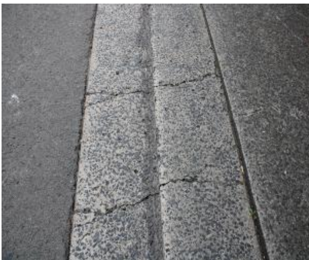
Figure 479 - Crack propagation through driveway layback and gutter heading North
