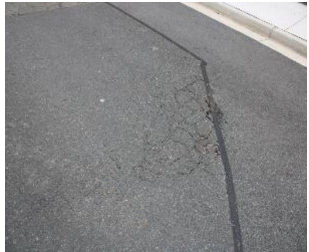
Figure 604 - Crack propagation through road surface heading South
