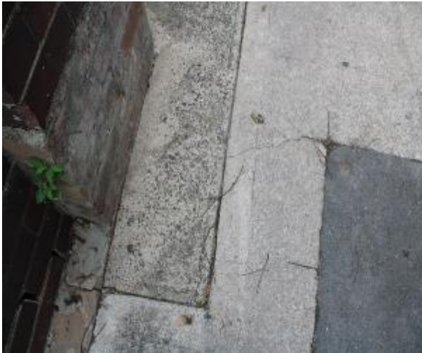
Figure 253 - Crack propagation through footpath pavement heading West
