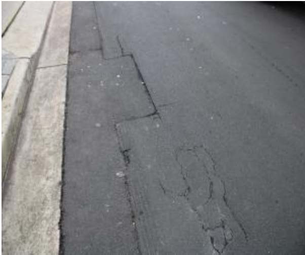
Figure 163 - Crack propagation through road surface heading East
