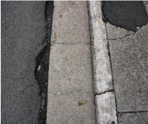
Figure 493 - Crack propagation through kerb and gutter heading North
