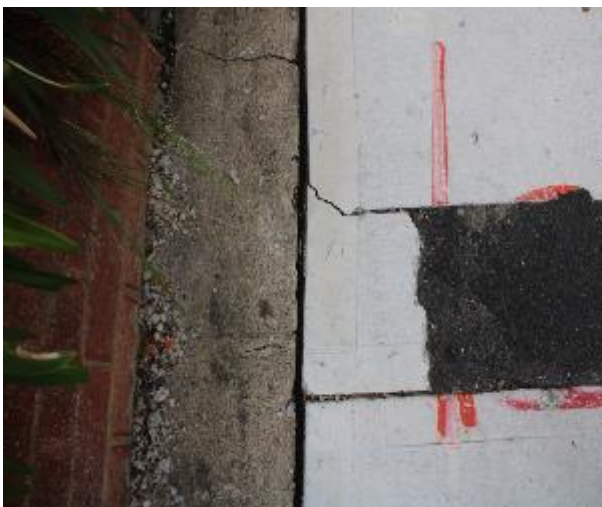
Figure 407 - Crack propagation through footpath pavement heading South
