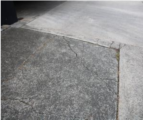
Figure 283 - Crack propagation through footpath pavement heading West
