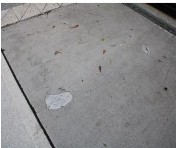
Figure 533 - Crack propagation through footpath pavement heading South
