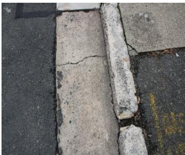
Figure 503 - Crack propagation and loss of material loss through kerb and gutter heading North
