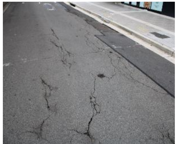
Figure 628 - Crack propagation through road surface heading South
