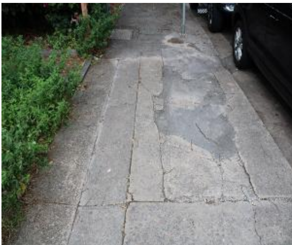
Figure 261 - Crack propagation through footpath pavement heading West
