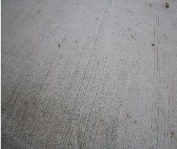
Figure 21 - Crack propagation through driveway pavement heading East
