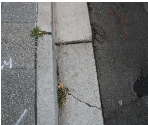
Figure 563 - Crack propagation through kerb and gutter heading North
