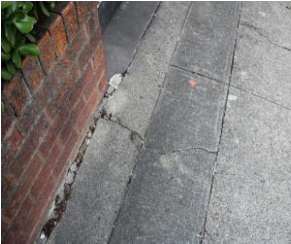
Figure 421 - Crack propagation through footpath pavement heading South
