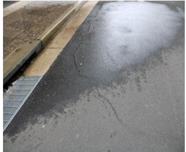
Figure 152 - Crack propagation through road surface heading East
