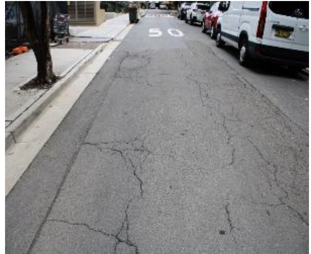
Figure 206 - Crack propagation through road surface heading East
