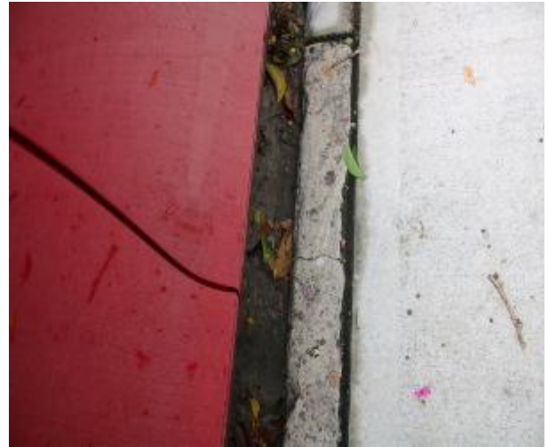
Figure 362 - Crack propagation through kerb and gutter heading East
