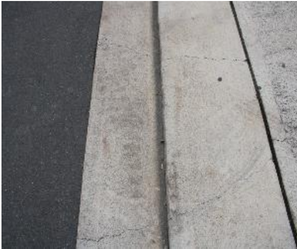
Figure 325 - Crack propagation through driveway layback and gutter heading East
