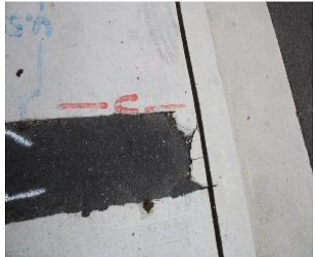
Figure 406 - Crack propagation through footpath pavement heading South
