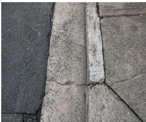
Figure 501 - Crack propagation and loss of materials through kerb and gutter heading North
