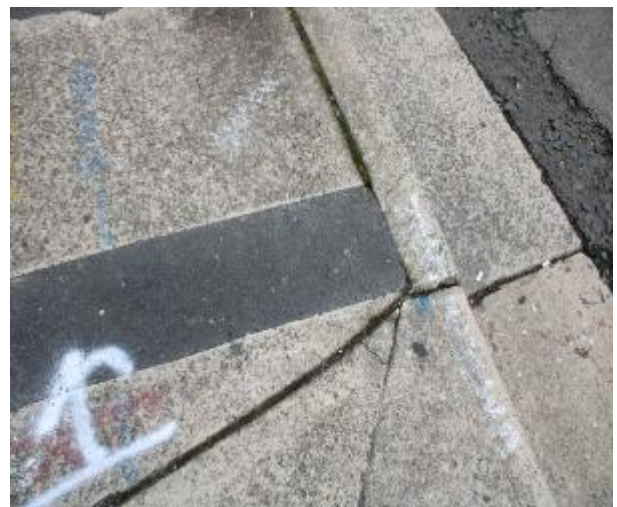
Figure 432 - Crack propagation and patchwork evident through footpath pavement heading South
