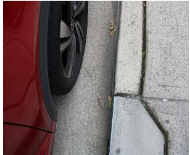
Figure 320 - Crack propagation through kerb and gutter heading East
