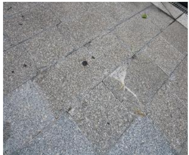
Figure 538 - Crack propagation through footpath pavers heading South
