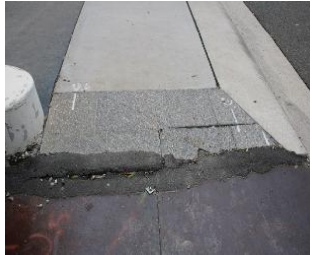
Figure 86 - Crack propagation through footpath pavement heading East
