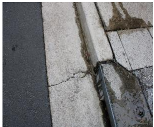
Figure 138 - Crack propagation through kerb and gutter heading West
