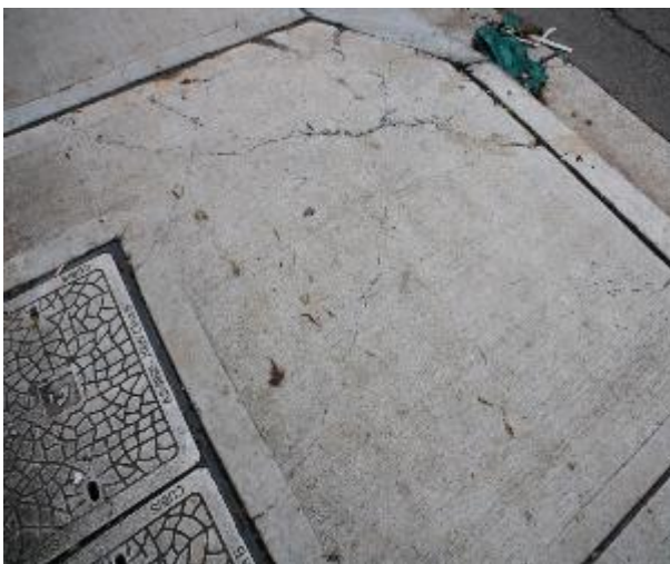
Figure 71 - Crack propagation through footpath pavement heading East
