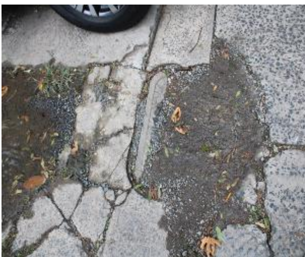
Figure 257 - Crack propagation and loss of materials through footpath pavement heading West
