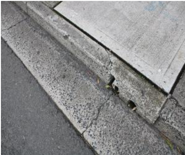
Figure 471 - Crack propagation through kerb and gutter heading North
