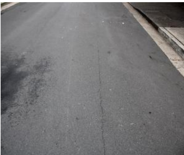
Figure 155 - Crack propagation through road surface heading East
