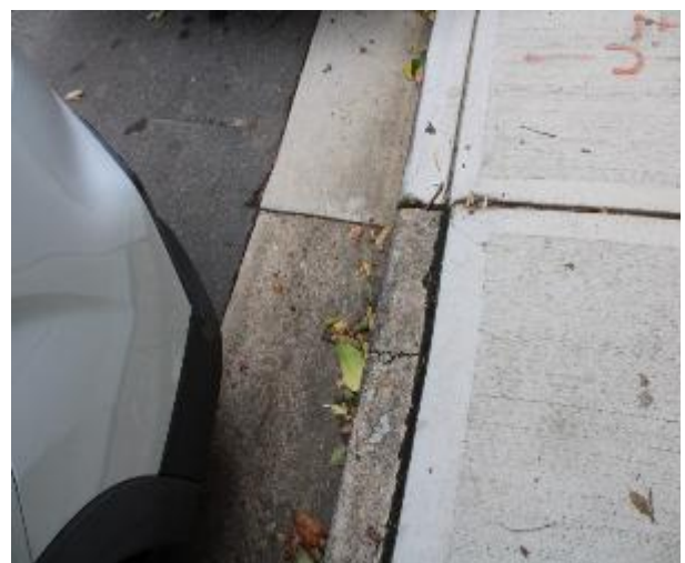
Figure 360 - Crack propagation through kerb and gutter heading East
