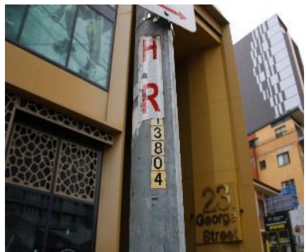
Figure 378 - General condition of street light post Identification No. HR13804
