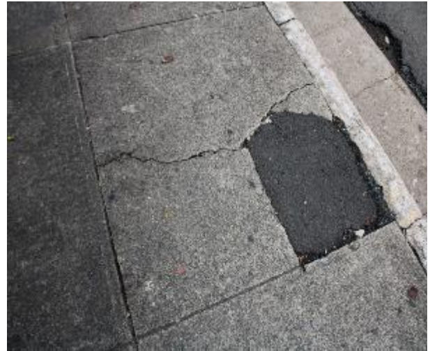
Figure 422 - Crack propagation and patchwork through footpath pavement heading South
