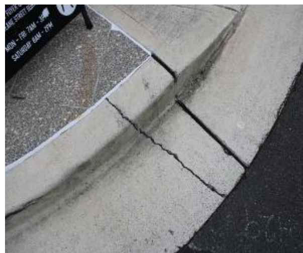
Figure 556 - Crack propagation through kerb and gutter heading North
