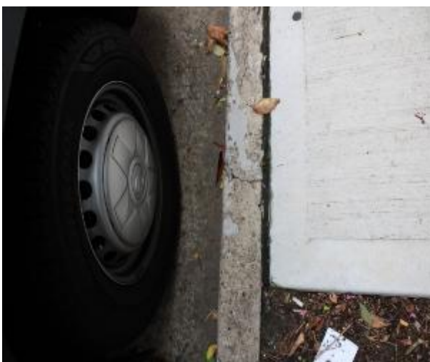
Figure 359 - Crack propagation through kerb and gutter heading East
