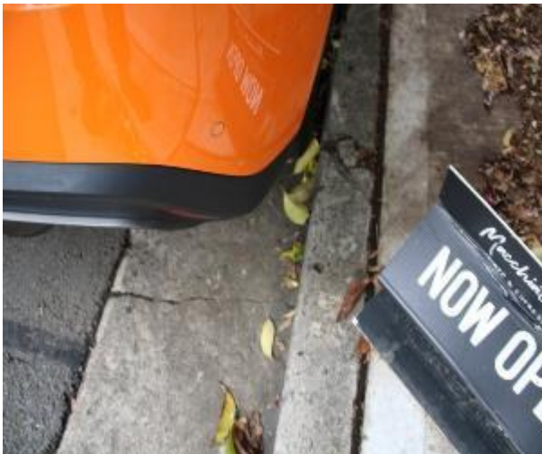
Figure 345 - Crack propagation through kerb and gutter heading East
