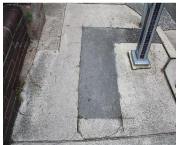
Figure 252 - General condition of patchwork evident through footpath pavement heading West
