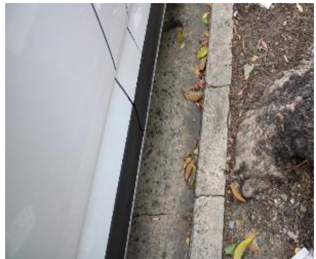
Figure 358 - Crack propagation through kerb and gutter heading East
