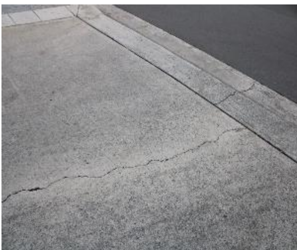
Figure 287 - Crack propagation through footpath pavement heading West
