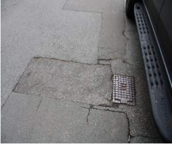
Figure 175 - Crack propagation and patchwork evident through road surface heading East
