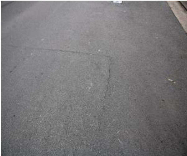
Figure 157 - Crack propagation through road surface heading East
