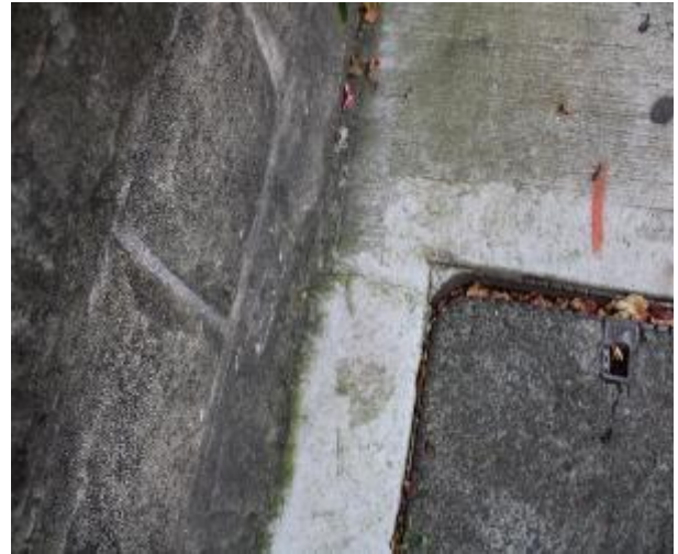
Figure 62 - Crack propagation through footpath pavement heading East
