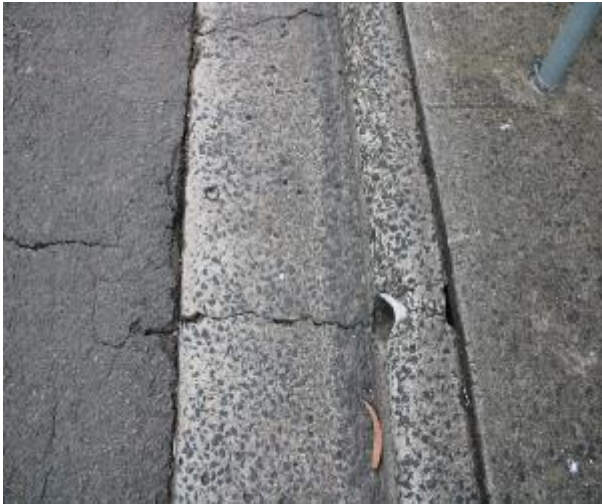
Figure 475 - Crack propagation through kerb and gutter heading North
