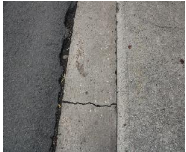
Figure 488 - Crack propagation through kerb and gutter heading North
