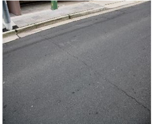
Figure 158 - Crack propagation through road surface heading East
