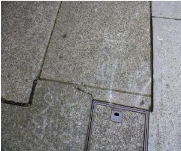
Figure 445 - Crack propagation through footpath pavement heading South
