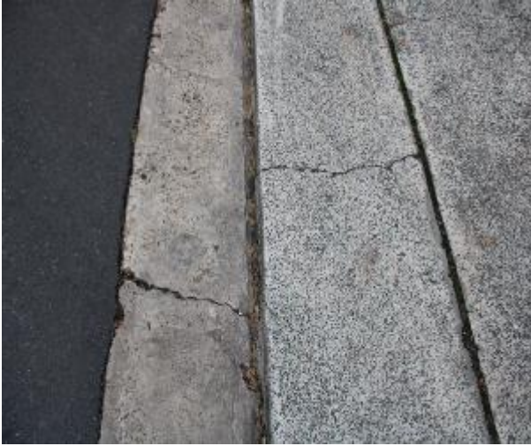
Figure 295 - Crack propagation through driveway layback and gutter heading East
