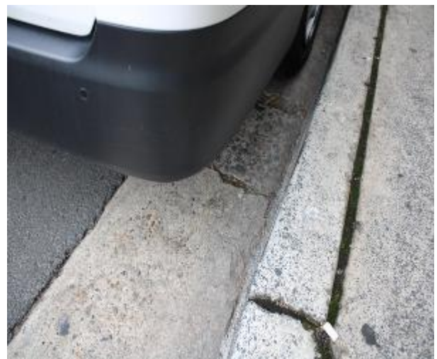
Figure 300 - Crack propagation through kerb and gutter heading East
