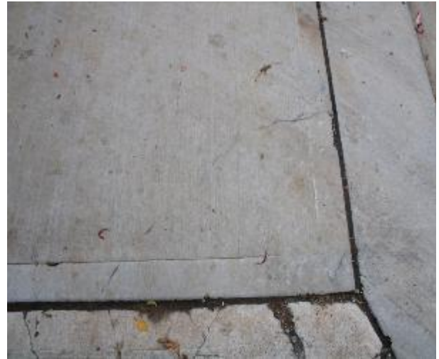
Figure 74 - Crack propagation through footpath pavement heading East
