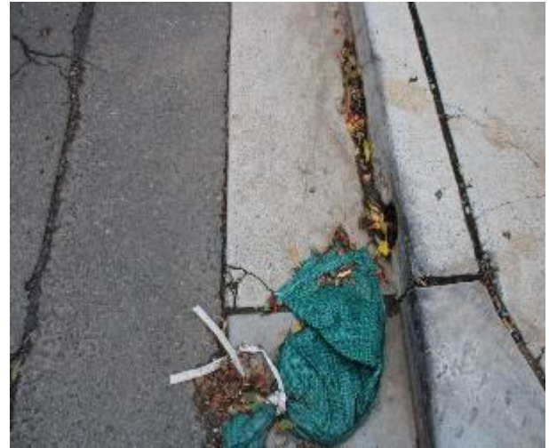
Figure 98 - Crack propagation through kerb and gutter heading West
