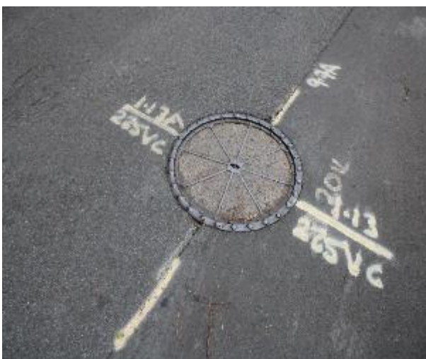
Figure 173 - General condition of sewer manhole cover
