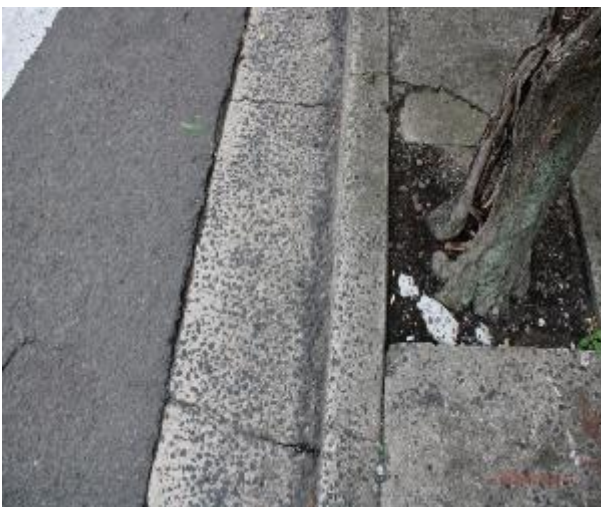
Figure 467 - Crack propagation through kerb and gutter heading North
