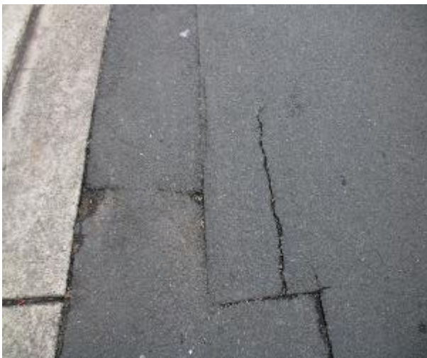
Figure 165 - Loss of material through road surface heading East
