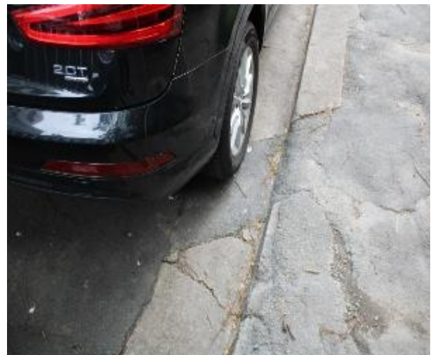
Figure 310 - Crack propagation through kerb and gutter heading East
