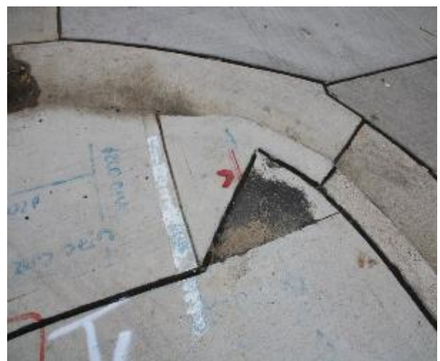
Figure 228 - Patchwork evident through footpath pavement heading West
