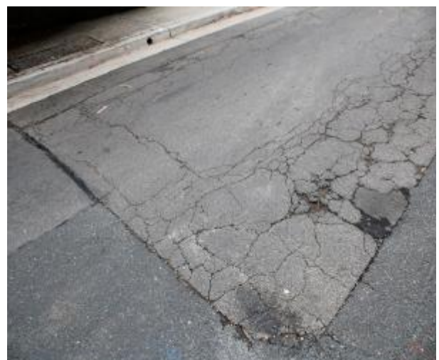
Figure 198 - Crack propagation and loss of materials through road surface heading East
