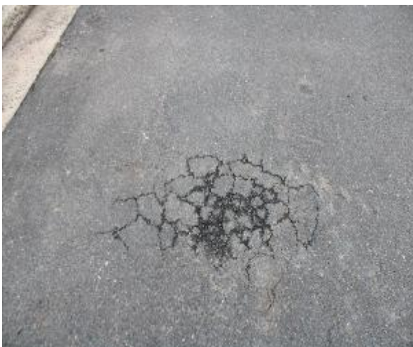
Figure 605 - Crack propagation through road surface heading South
