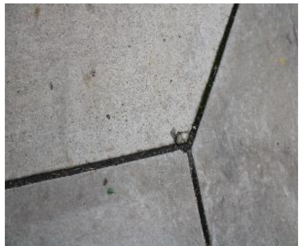
Figure 48 - Crack propagation through footpath pavement heading East
