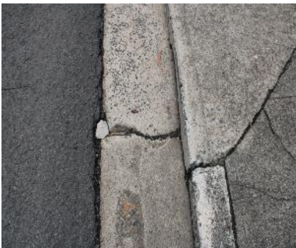
Figure 497 - Loss of material through driveway layback and gutter heading North
