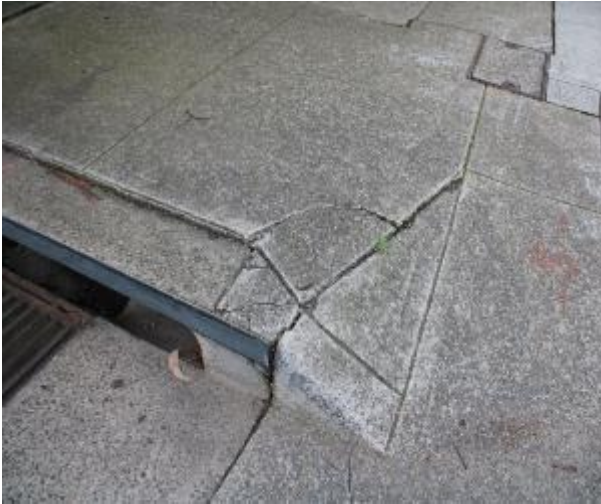
Figure 441 - Crack propagation through footpath pavement heading South
