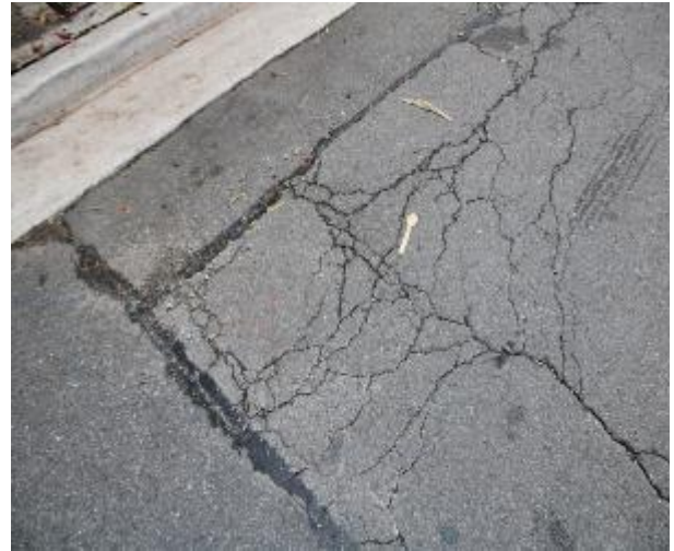
Figure 200 - Crack propagation through road surface heading East
