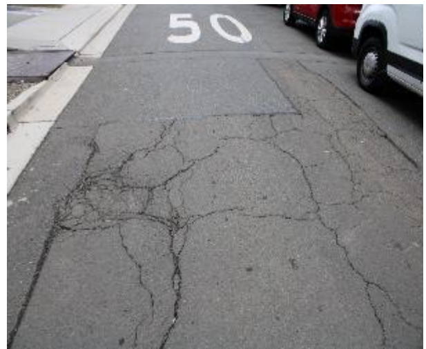
Figure 208 - Crack propagation through road surface heading East
