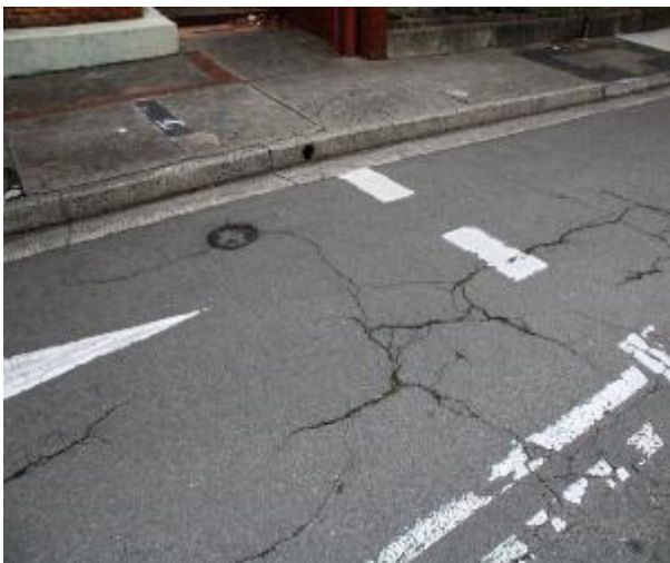
Figure 639 - Crack propagation through road surface heading South
