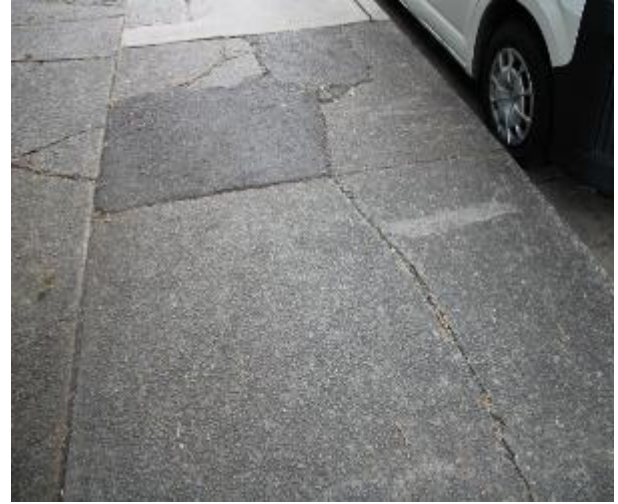
Figure 272 - Crack propagation through footpath pavement heading West
