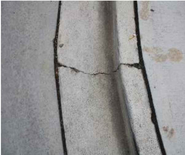
Figure 337 - Crack propagation through kerb and gutter heading East
