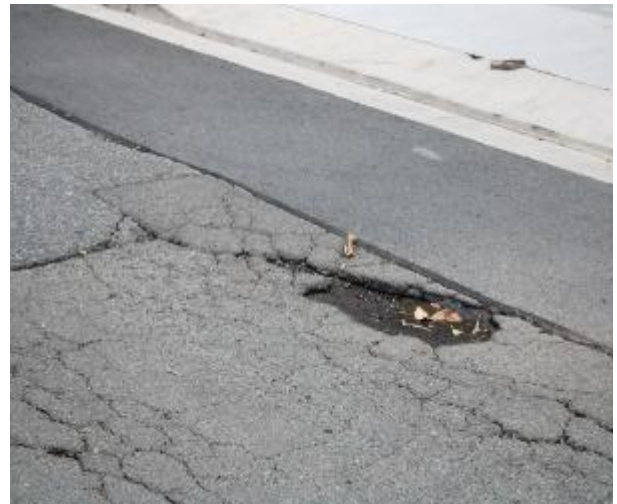
Figure 622 - Crack propagation and loss of materials through road surface heading South
