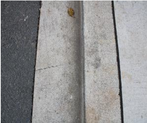
Figure 343 - Crack propagation through kerb and gutter heading East
