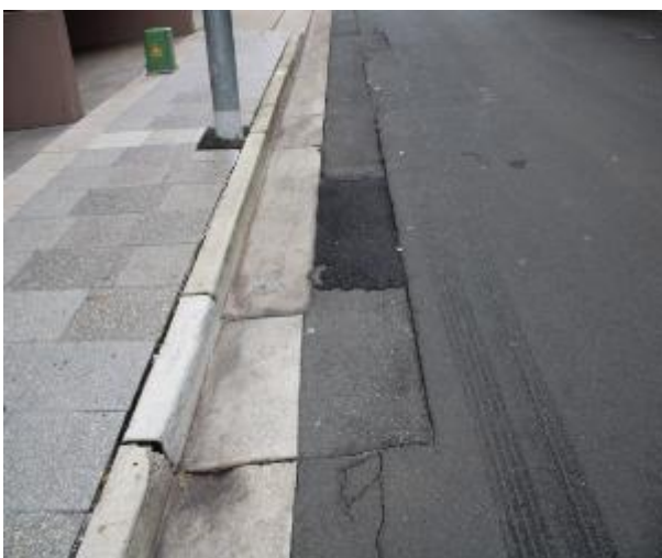
Figure 161 - Patchwork evident through road surface heading East
