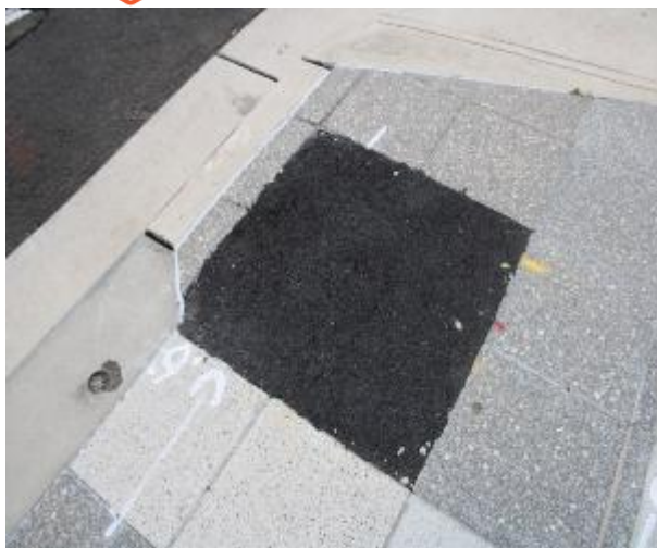
Figure 553 - Patchwork evident through footpath pavers heading South
