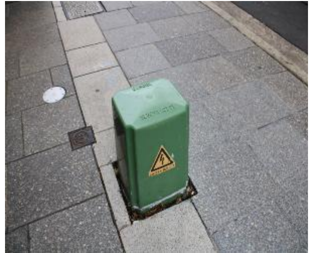
Figure 386 - General condition of electricity box identification No. 36361
