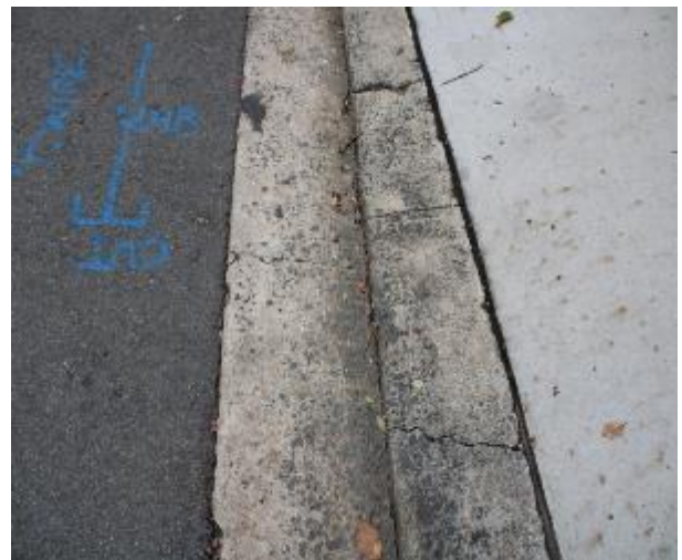
Figure 352 - Crack propagation through driveway layback and gutter heading East
