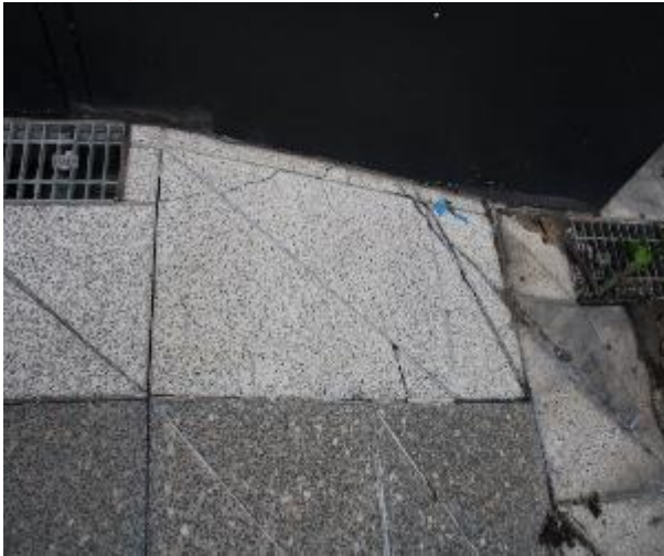
Figure 541 - Crack propagation through footpath pavers heading South
