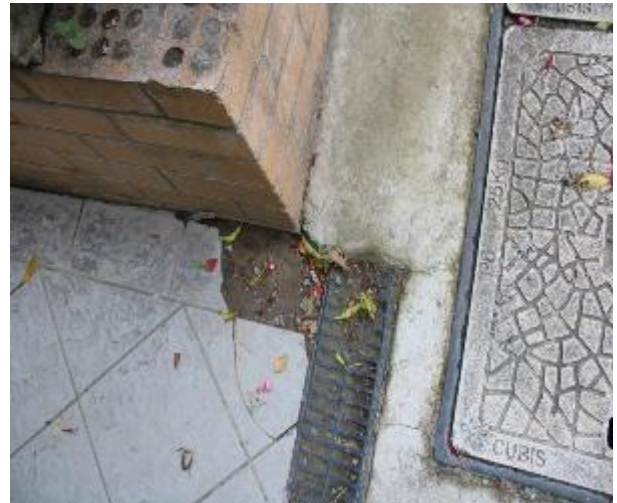
Figure 70 - Crack propagation through footpath pavement heading East
