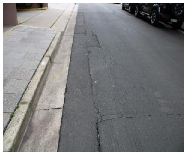
Figure 162 - Crack propagation through road surface heading East
