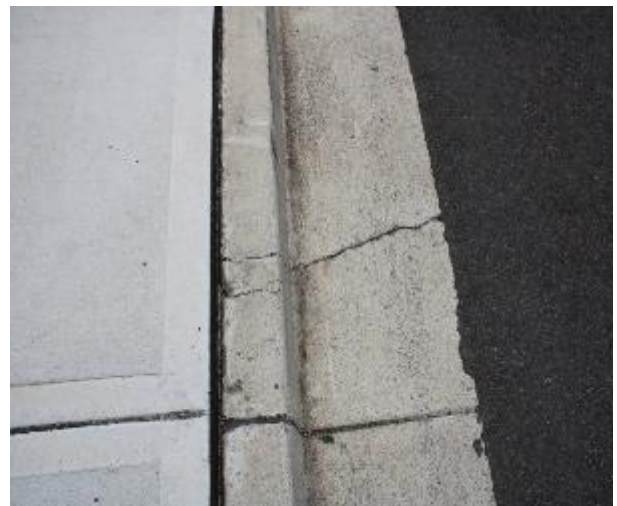
Figure 580 - Crack propagation through kerb and gutter heading North
