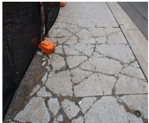
Figure 78 - Crack propagation through footpath pavement heading East
