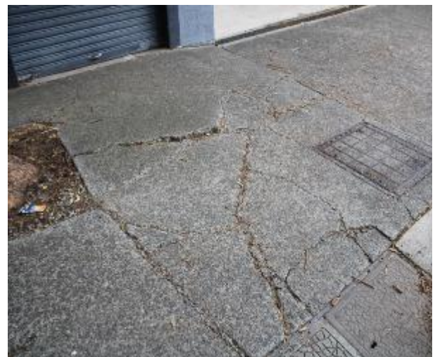
Figure 276 - Crack propagation through footpath pavement heading West
