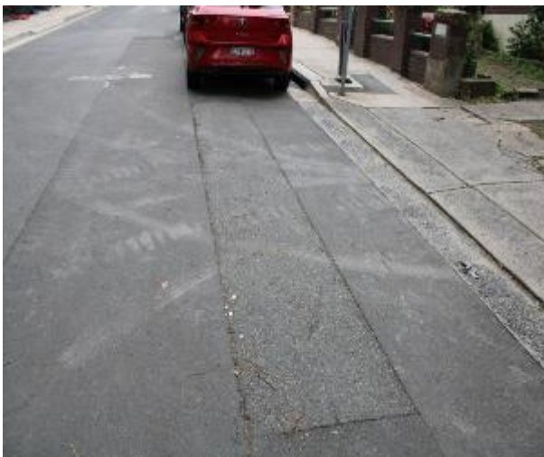
Figure 171 - Patchwork evident through road surface heading East
