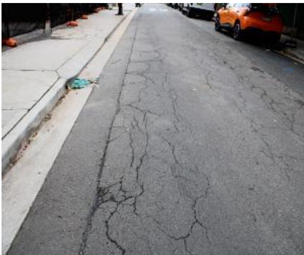
Figure 201 - Crack propagation through road surface heading East
