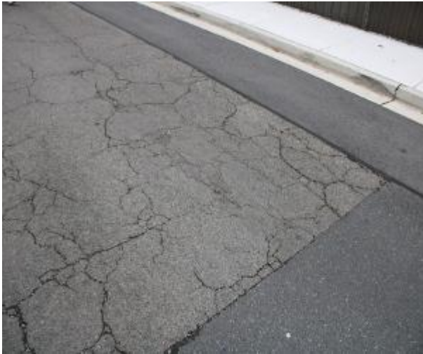
Figure 607 - Crack propagation through road surface heading South
