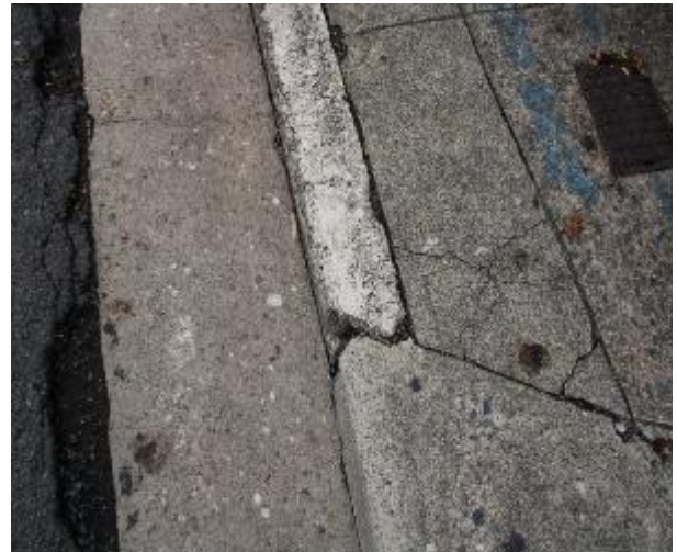
Figure 490 - Loss of material through kerb and gutter heading North
