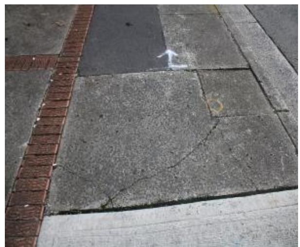
Figure 456 - Crack propagation through footpath pavement heading South
