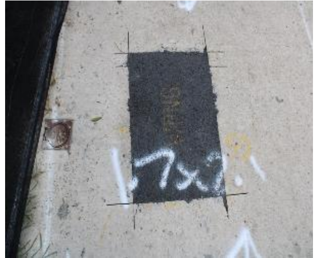
Figure 40 - Patchwork evident through footpath pavement heading East
