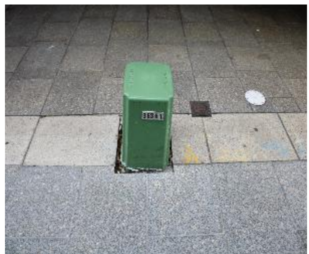
Figure 384 - General condition of electricity box identification No. 36361
