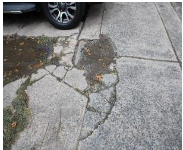
Figure 256 - Crack propagation and loss of materials through footpath pavement heading West
