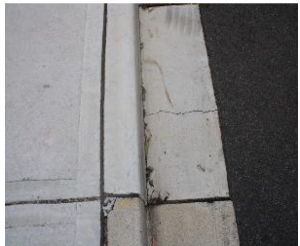
Figure 588 - Crack propagation through kerb and gutter heading North
