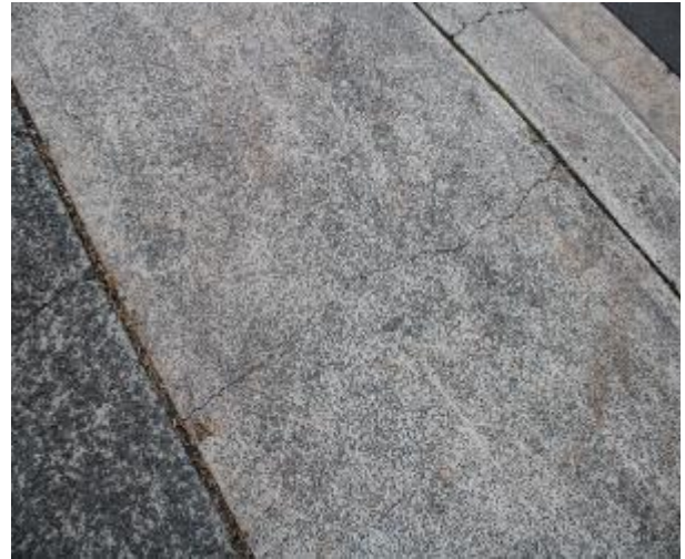
Figure 284 - Crack propagation through footpath pavement heading West
