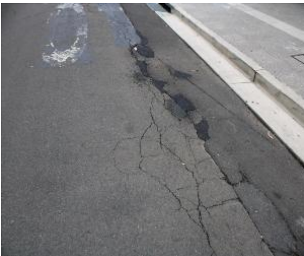
Figure 633 - Crack propagation through road surface heading South
