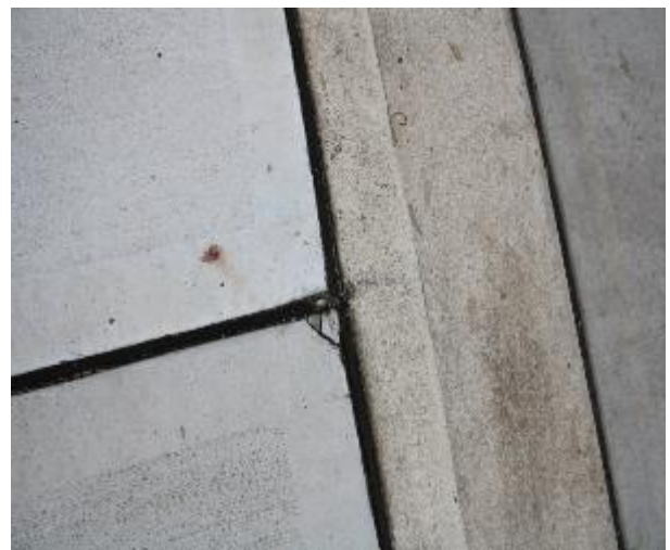
Figure 402 - Crack propagation through footpath pavement heading South
