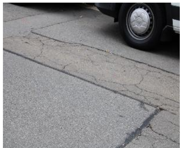
Figure 210 - Crack propagation through road surface heading East
