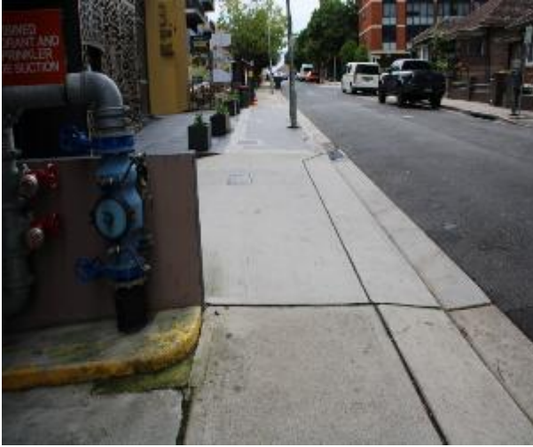
Figure 19 - General condition of driveway pavement heading East
