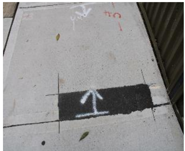
Figure 522 - Patchwork evident through footpath pavement heading South
