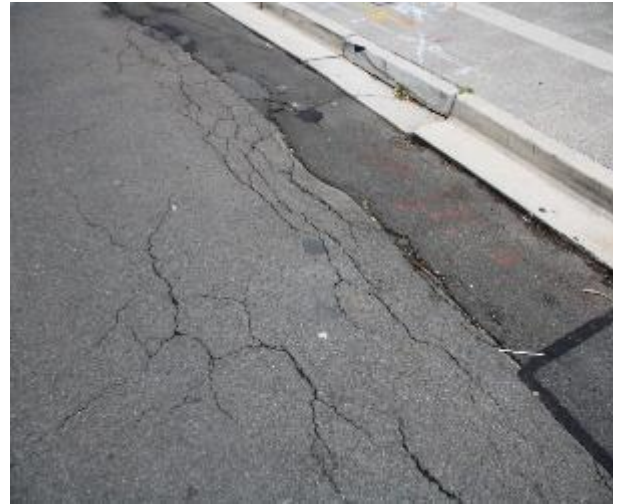
Figure 632 - Crack propagation and patchwork through road surface heading South
