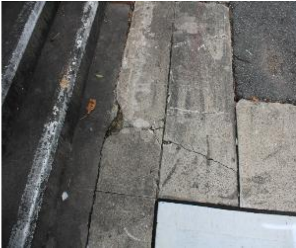
Figure 409 - Crack propagation and loss of materials through footpath pavement heading South
