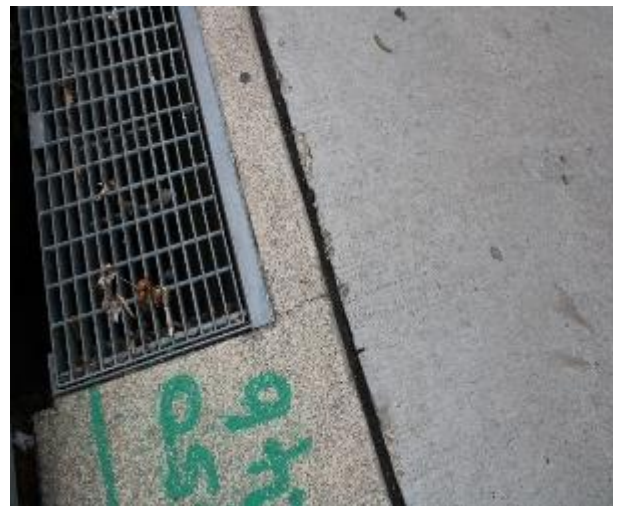
Figure 592 - Crack propagation through kerb and gutter heading North
