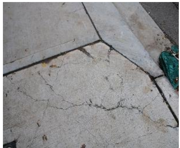
Figure 72 - Crack propagation through footpath pavement heading East
