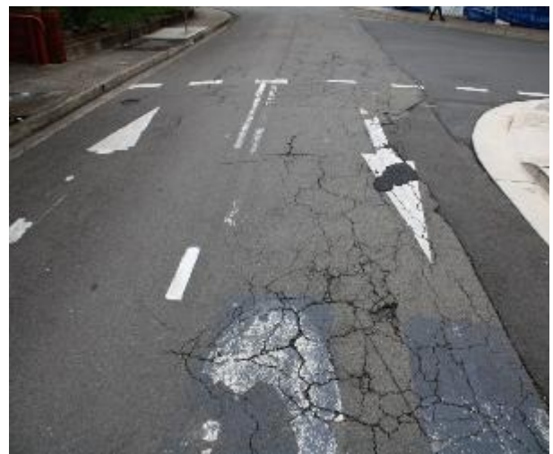
Figure 636 - Crack propagation through road surface heading South
