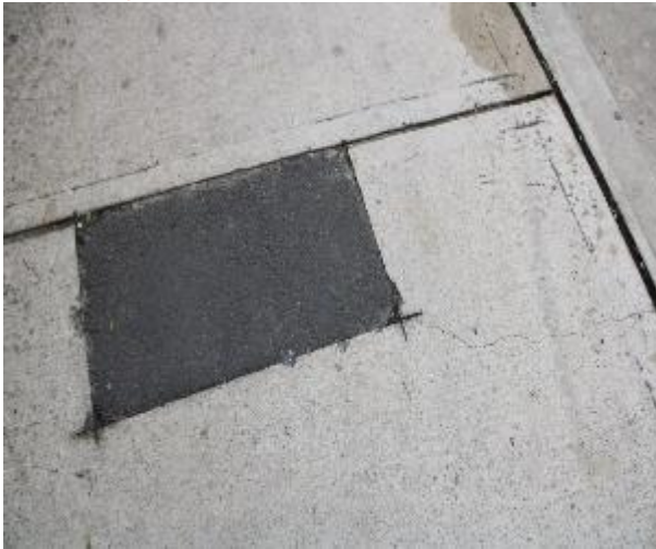
Figure 49 - Crack propagation and patchwork evident through footpath pavement heading East
