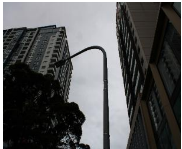
Figure 382 - General condition of street light post Identification No. HR13804
