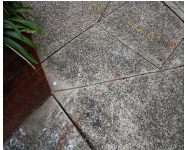
Figure 436 - Crack propagation through footpath pavement heading South
