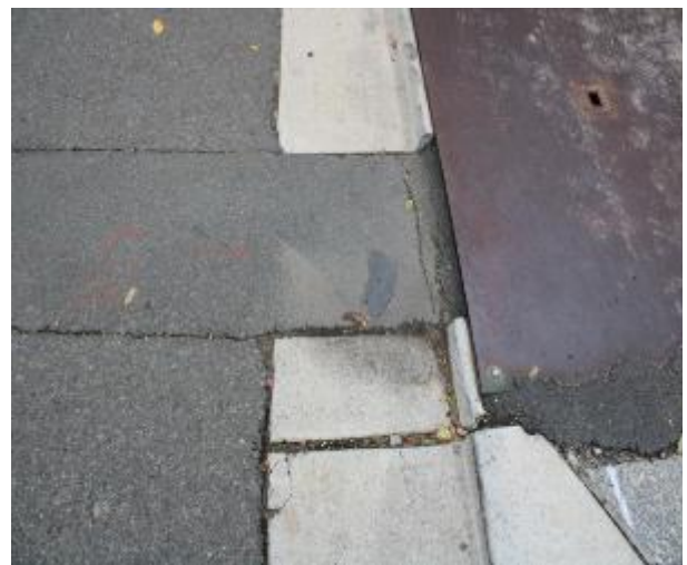
Figure 90 - Crack propagation through kerb and gutter heading West
