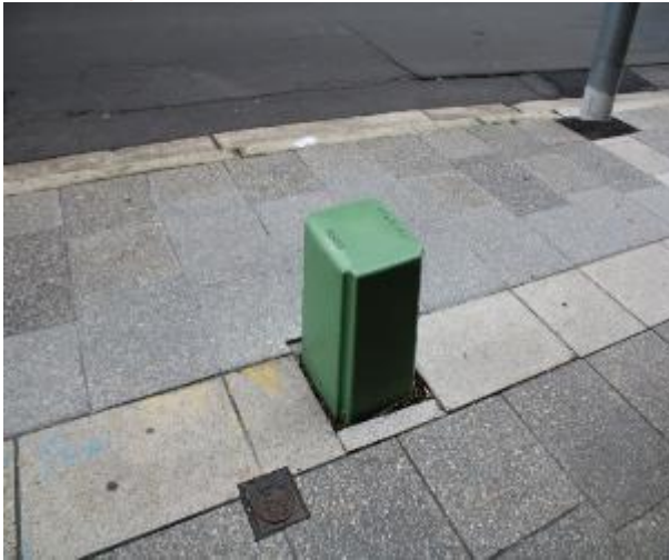
Figure 385 - General condition of electricity box identification No. 36361
