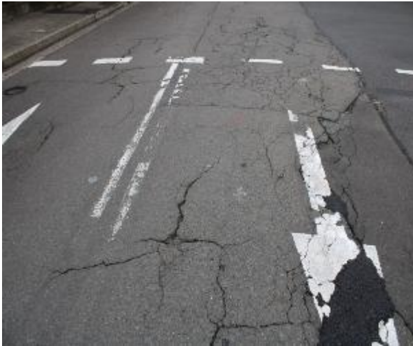
Figure 637 - Crack propagation through road surface heading South
