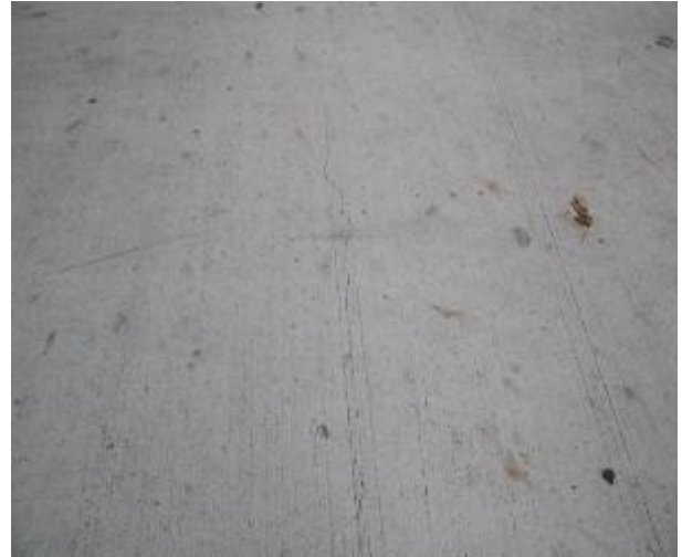
Figure 22 - Crack propagation through driveway pavement heading East
