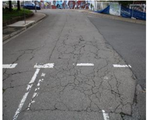
Figure 638 - Crack propagation through road surface heading South
