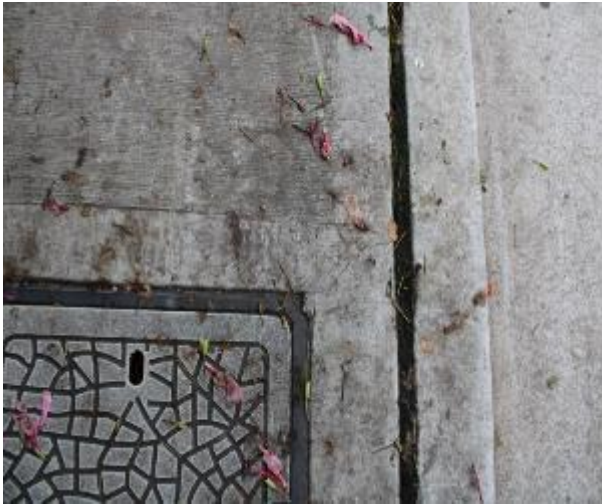
Figure 67 - Crack propagation through footpath pavement heading East
