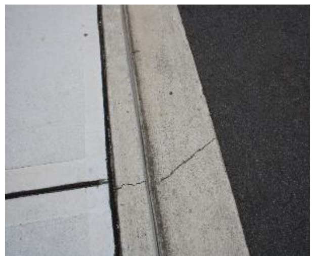
Figure 582 - Crack propagation through kerb and gutter heading North
