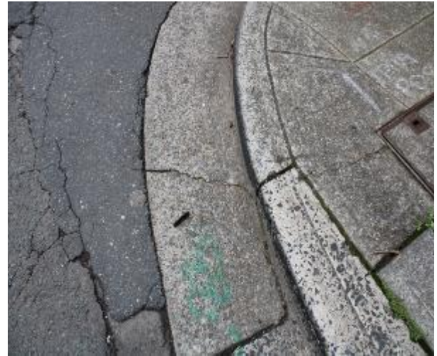
Figure 482 - Crack propagation through kerb and gutter heading North
