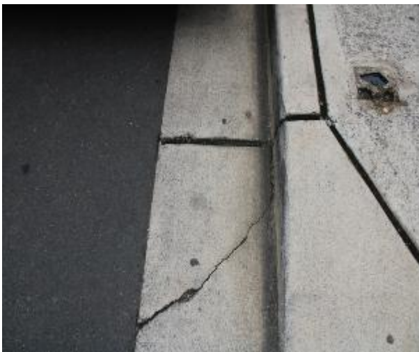
Figure 327 - Crack propagation through kerb and gutter heading East
