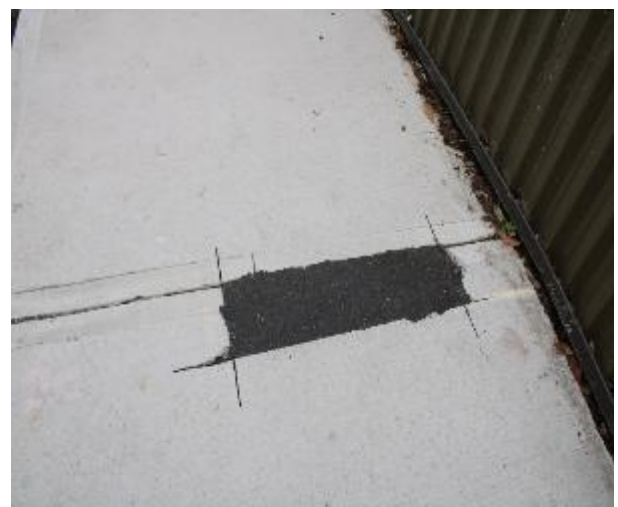
Figure 516 - Patchwork evident through footpath pavement heading South
