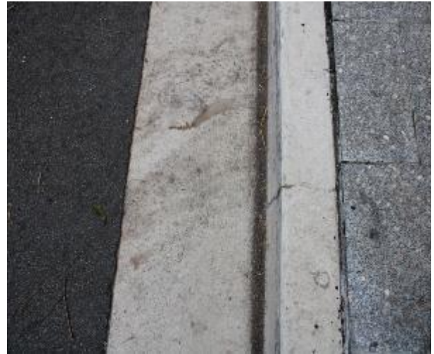
Figure 122 - Crack propagation through kerb and gutter heading West
