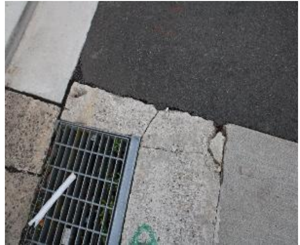
Figure 602 - Crack propagation and loss of materials through road surface heading South
