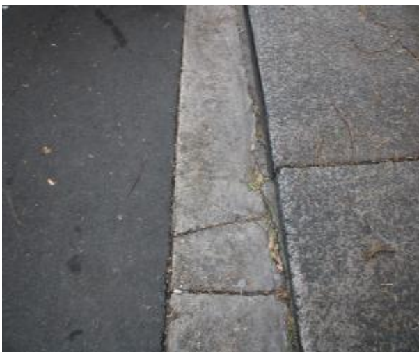
Figure 305 - Crack propagation through kerb and gutter heading East
