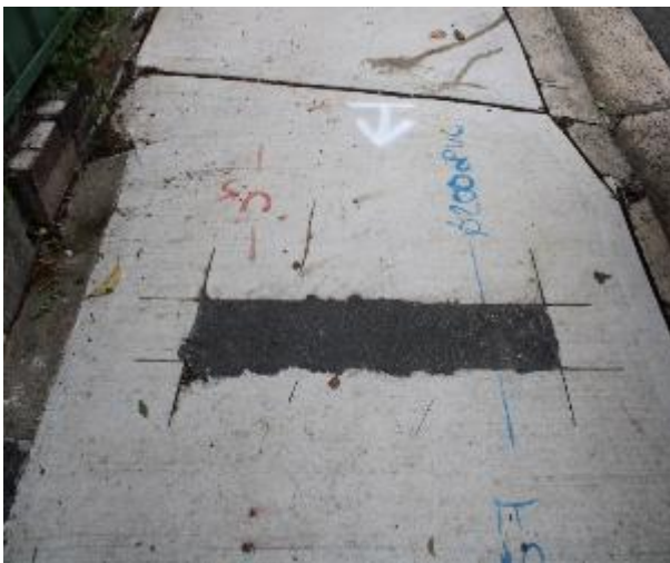
Figure 219 - Patchwork evident through footpath pavement heading West
