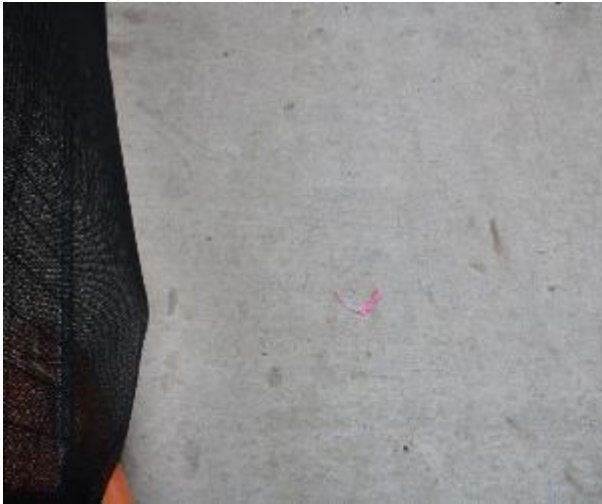
Figure 43 - Crack propagation through driveway pavement heading East
