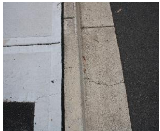
Figure 574 - Crack propagation through kerb and gutter heading North
