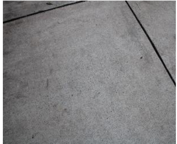
Figure 44 - Crack propagation through driveway pavement heading East
