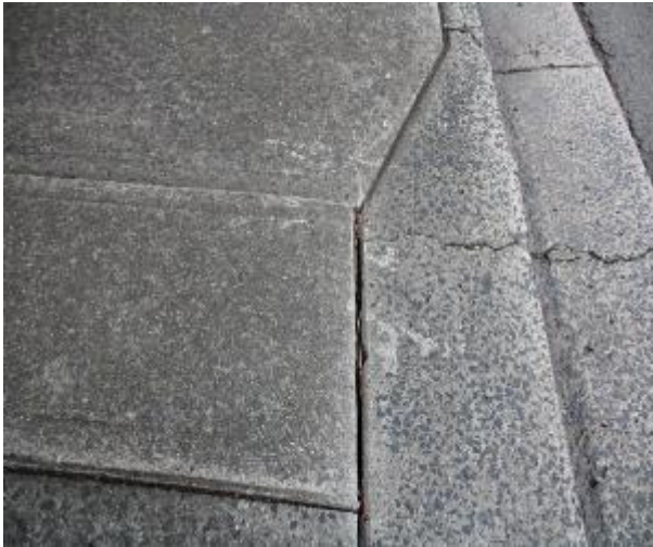
Figure 451 - Crack propagation through footpath pavement heading South
