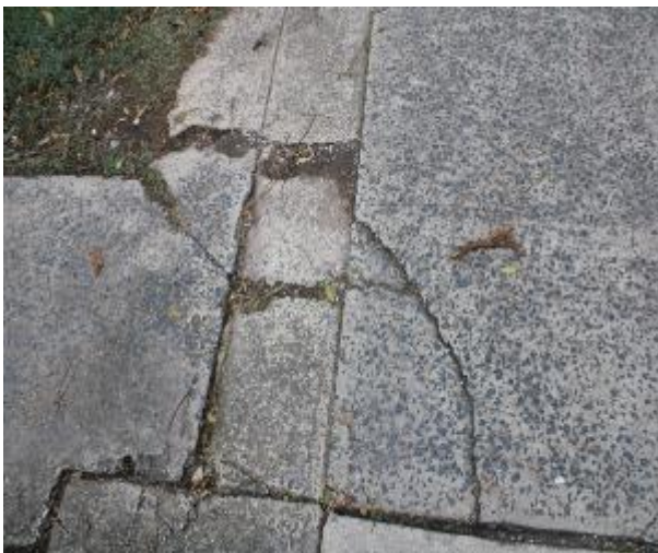
Figure 255 - Crack propagation through footpath pavement heading West
