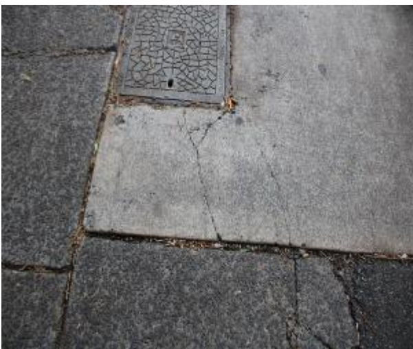
Figure 275 - Crack propagation through footpath pavement heading West
