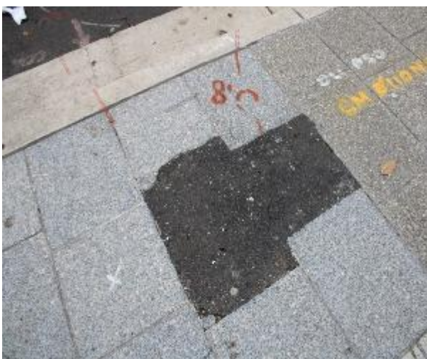
Figure 545 - Patchwork evident through footpath pavers heading South
