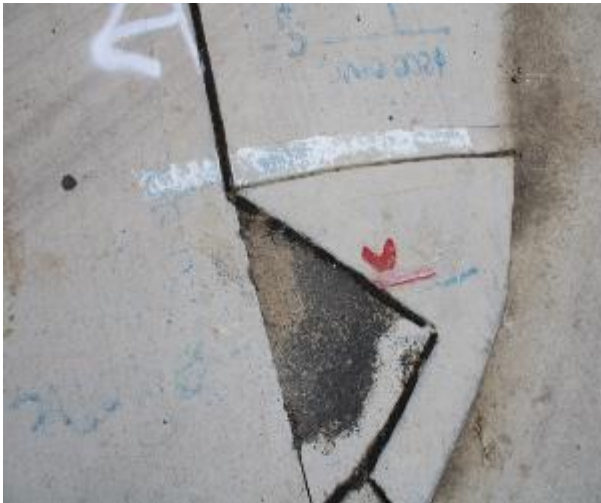
Figure 399 - Patchwork evident through footpath pavement heading South
