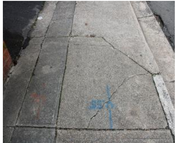
Figure 412 - Crack propagation through footpath pavement heading South
