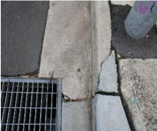
Figure 109 - Crack propagation through kerb and gutter heading West
