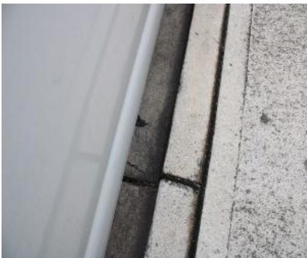
Figure 329 - Crack propagation through kerb and gutter heading East
