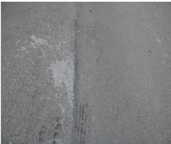
Figure 183 - Crack propagation through road surface heading East
