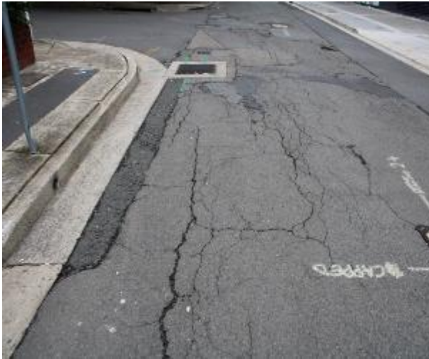
Figure 613 - Crack propagation through road surface heading South
