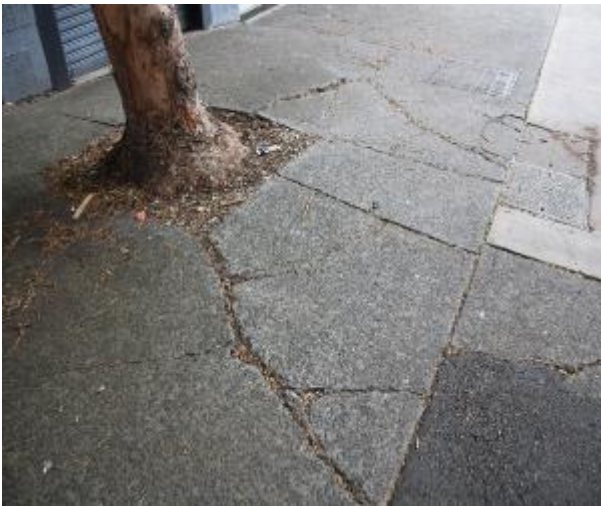
Figure 273 - Crack propagation through footpath pavement heading West
