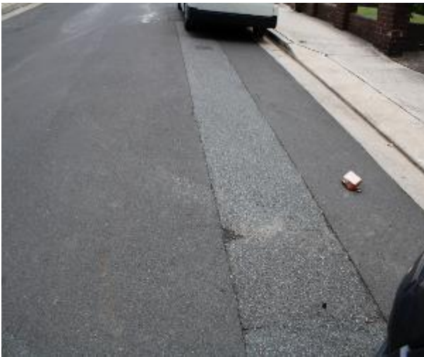
Figure 177 - Patchwork evident through road surface heading East
