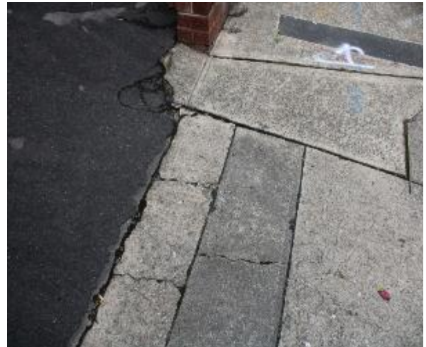
Figure 430 - Crack propagation through footpath pavement heading South
