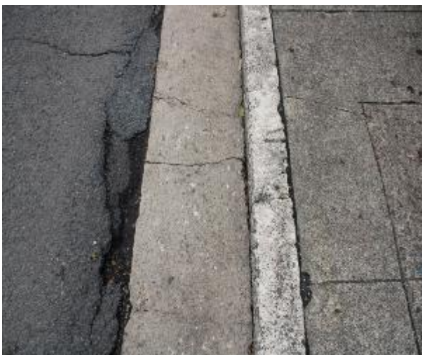
Figure 491 - Crack propagation through kerb and gutter heading North
