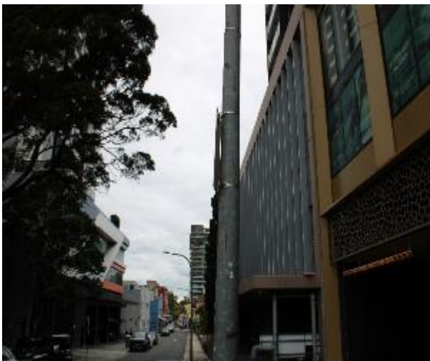
Figure 381 - General condition of street light post Identification No. HR13804
