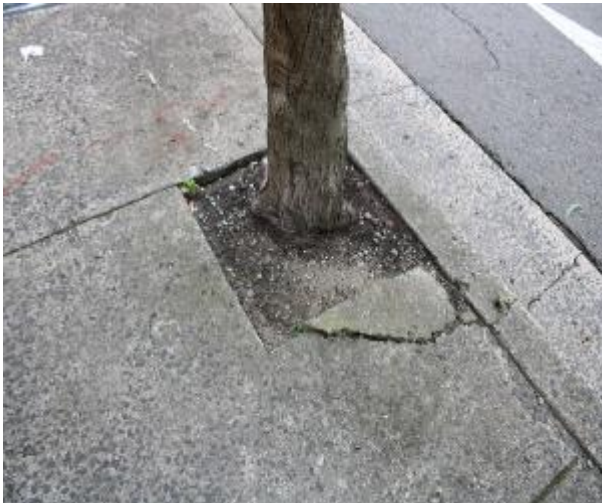
Figure 459 - Crack propagation through footpath pavement heading South
