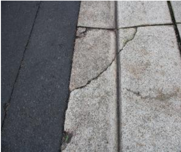
Figure 127 - Crack propagation through driveway layback and gutter heading West
