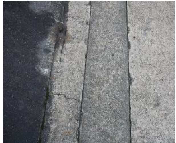
Figure 416 - Crack propagation through footpath pavement heading South
