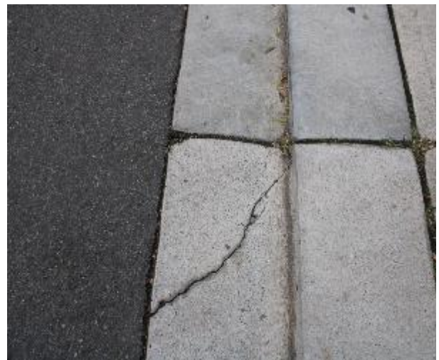
Figure 106 - Crack propagation through kerb and gutter heading West
