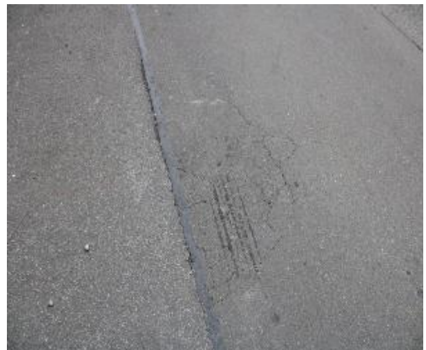
Figure 184 - Crack propagation through road surface heading East
