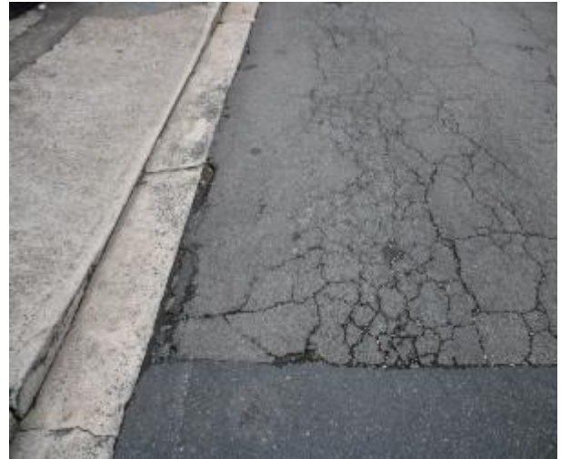
Figure 608 - Crack propagation through road surface heading South
