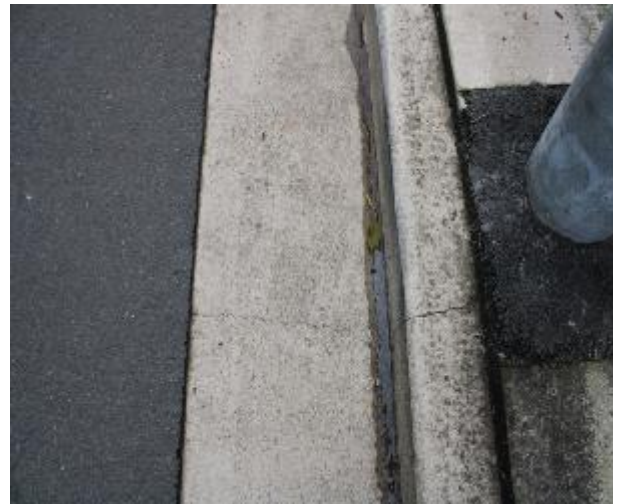
Figure 142 - Crack propagation through kerb and gutter heading West
