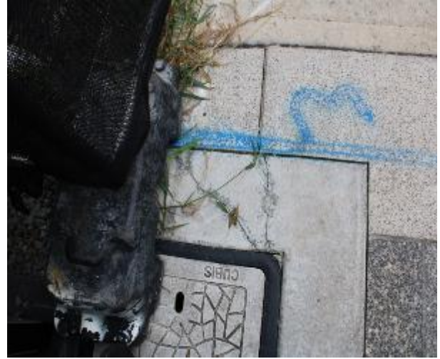
Figure 38 - Crack propagation through footpath pavers heading East
