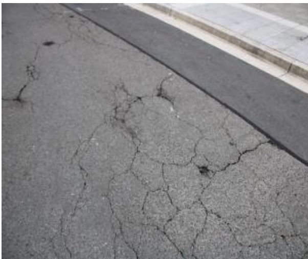
Figure 627 - Crack propagation through road surface heading South
