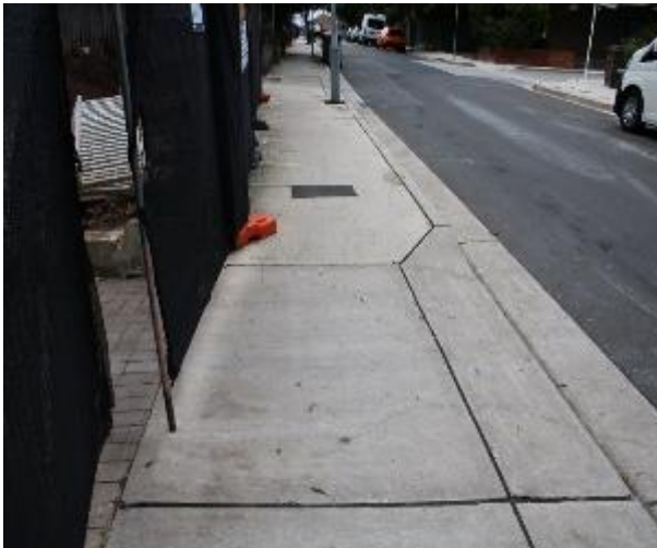
Figure 45 - General condition of driveway pavement heading East
