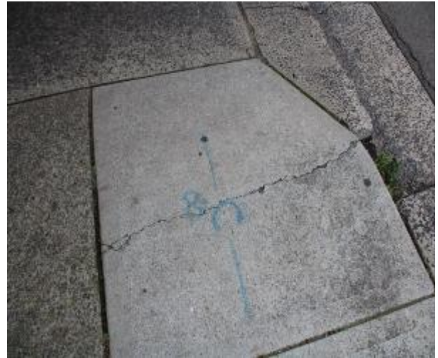
Figure 446 - Crack propagation through footpath pavement heading South
