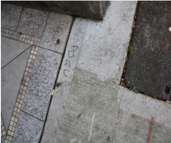
Figure 61 - Crack propagation through footpath pavement heading East
