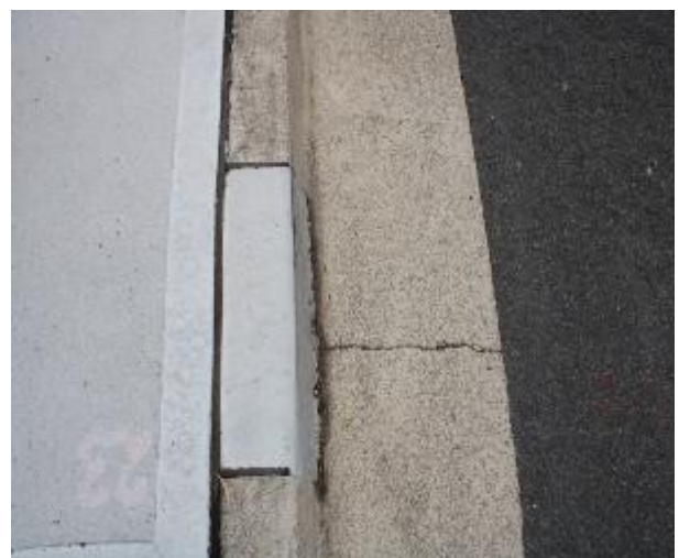
Figure 576 - Crack propagation through kerb and gutter heading North
