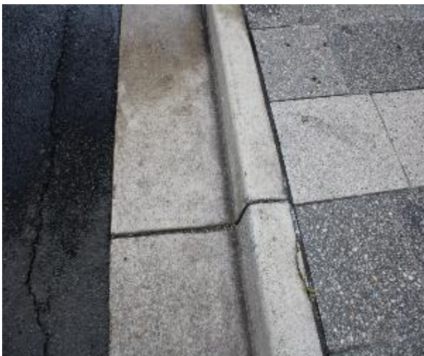
Figure 135 - Crack propagation through kerb and gutter heading West
