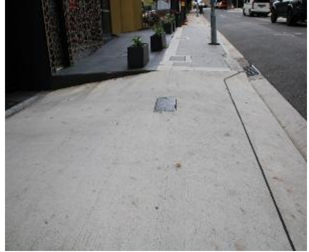
Figure 20 - General condition of driveway pavement heading East
