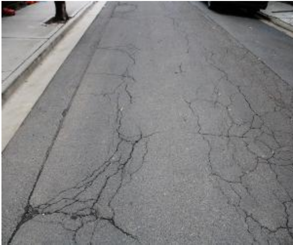
Figure 205 - Crack propagation through road surface heading East
