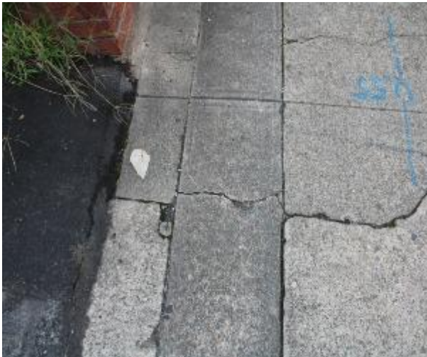
Figure 417 - Crack propagation through footpath pavement heading South
