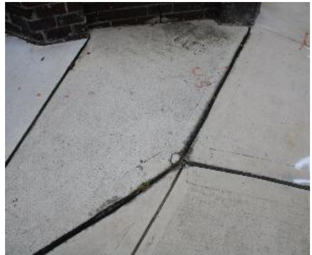
Figure 232 - Crack propagation through footpath pavement heading West
