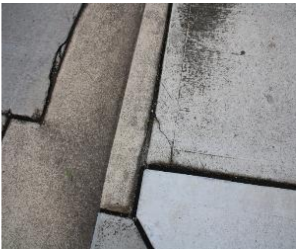
Figure 513 - Crack propagation through footpath pavement heading South
