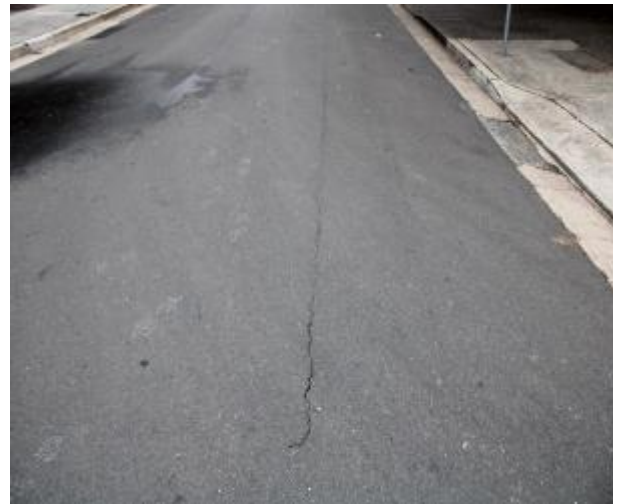
Figure 154 - Crack propagation through road surface heading East
