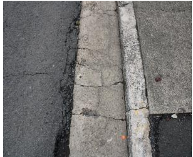
Figure 494 - Crack propagation through kerb and gutter heading North
