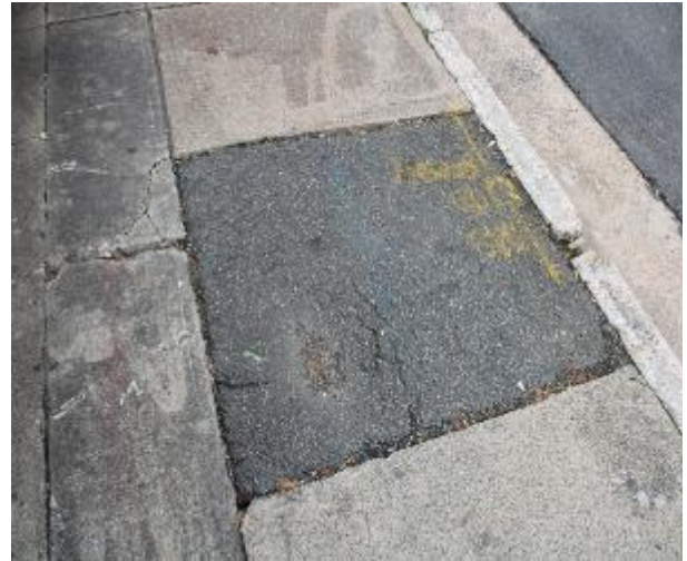
Figure 410 - Crack propagation and patchwork evident through footpath pavement heading South
