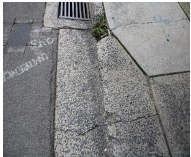
Figure 480 - Crack propagation through driveway layback and gutter heading North
