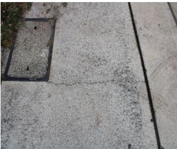
Figure 245 - Crack propagation through footpath pavement heading West
