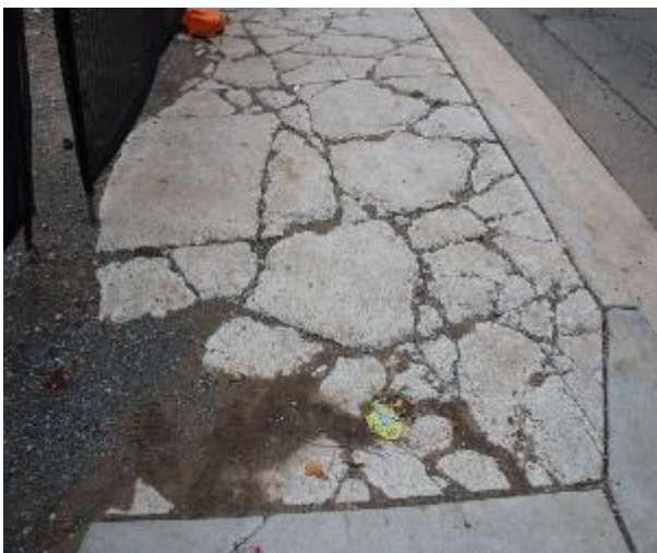
Figure 77 - Crack propagation and loss of materials through footpath pavement heading East
