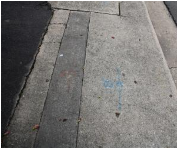
Figure 429 - Crack propagation through footpath pavement heading South
