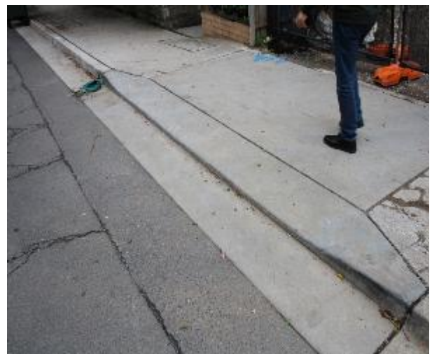
Figure 96 - General condition of driveway layback and gutter heading West
