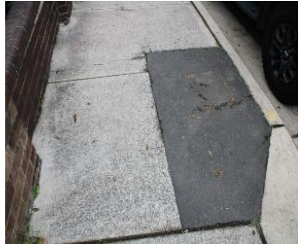
Figure 248 - Patchwork evident through footpath pavement heading West
