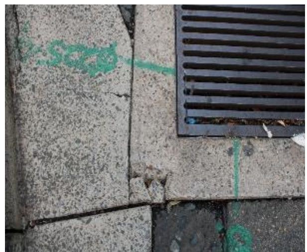
Figure 618 - Crack propagation and loss of materials through road surface heading South
