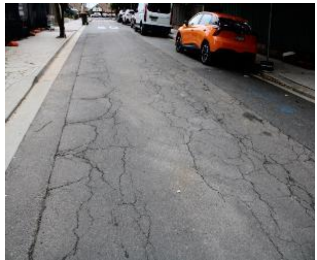
Figure 202 - Crack propagation through road surface heading East
