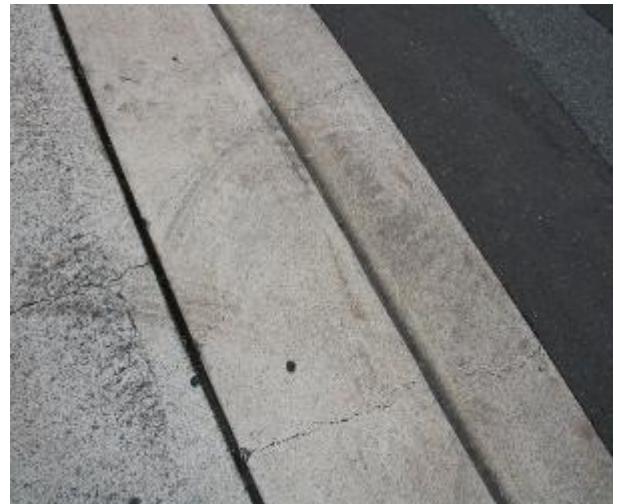
Figure 244 - Crack propagation through footpath pavement heading West
