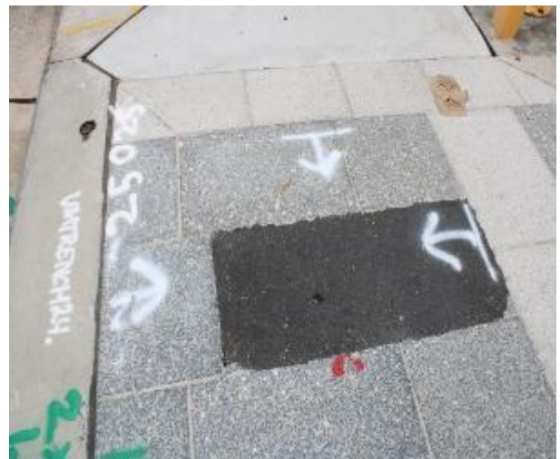
Figure 526 - Patchwork evident through footpath pavement heading South
