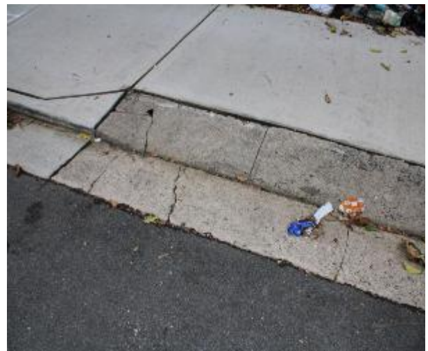
Figure 364 - Crack propagation through driveway layback and gutter heading East
