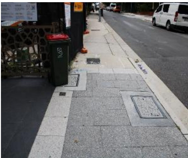
Figure 35 - General condition of footpath pavers heading East
