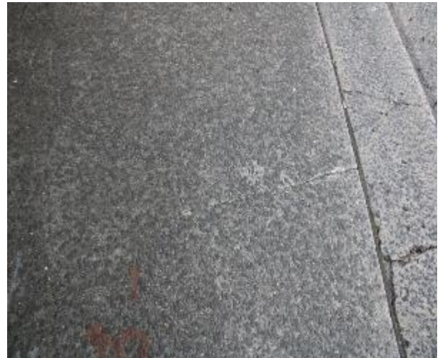
Figure 448 - Crack propagation through footpath pavement heading South
