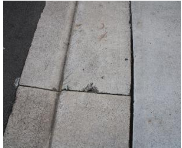
Figure 530 - Loss of material through footpath pavement heading South
