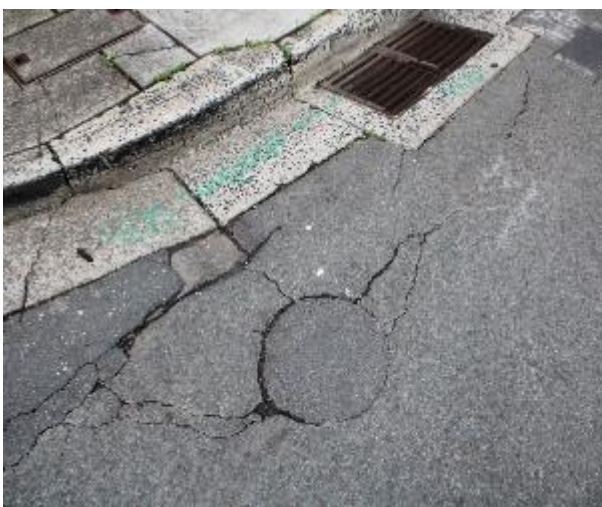
Figure 629 - Crack propagation through road surface heading South
