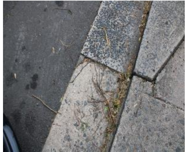
Figure 314 - Crack propagation through kerb and gutter heading East
