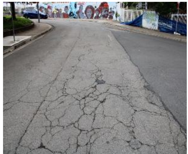
Figure 640 - Crack propagation through road surface heading South
