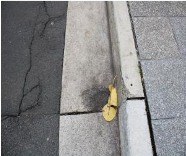
Figure 133 - Loss of material through kerb and gutter heading West
