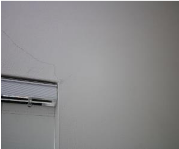
Figure 1068 - Crack propagation through bedroom 2 internal wall
