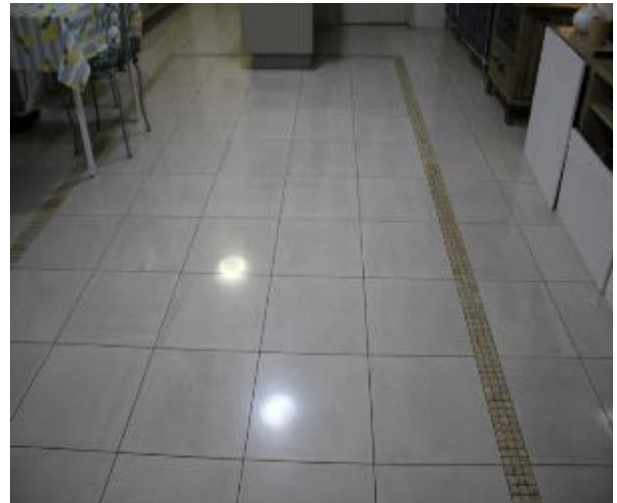
Figure 524 - General condition of open kitchen/ lounge room floor tiles
