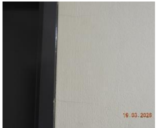
Figure 52 - Crack propagation through level 2 common area internal wall
