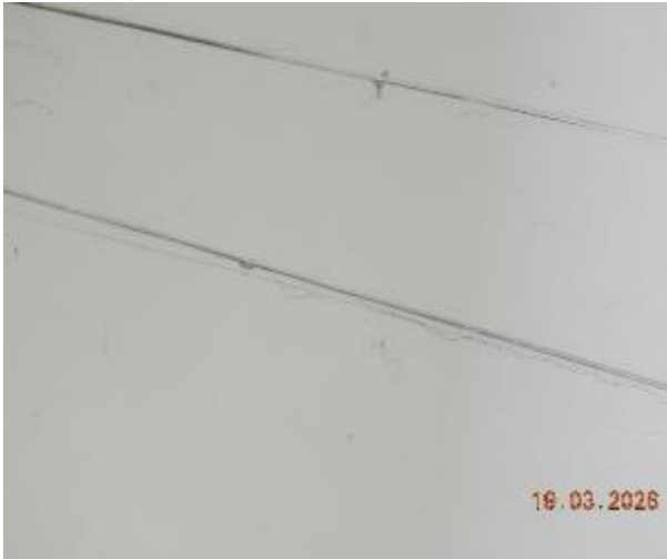
Figure 336 - Crack propagation through level 3 fire stairs internal wall
