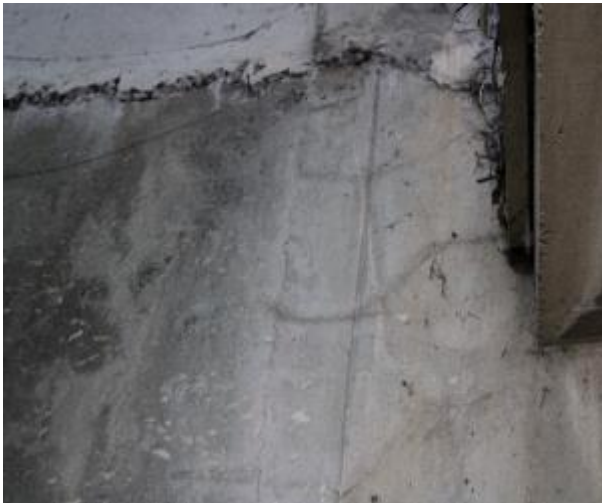
Figure 205 - Crack propagation through B2 fire stairs internal wall
