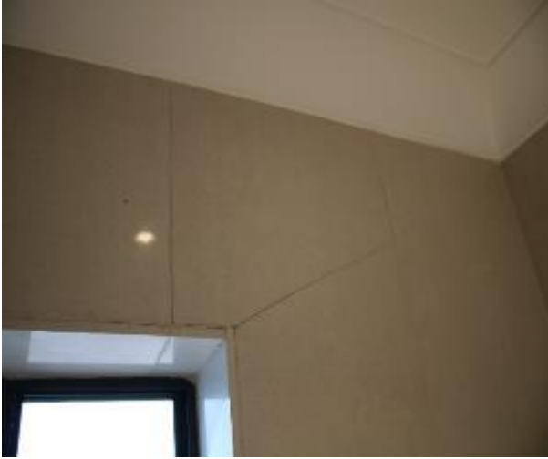
Figure 1002 - Crack propagation through bathroom 1 internal wall
