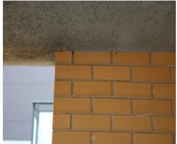
Figure 1449 - Crack propagation through balcony underside slab
