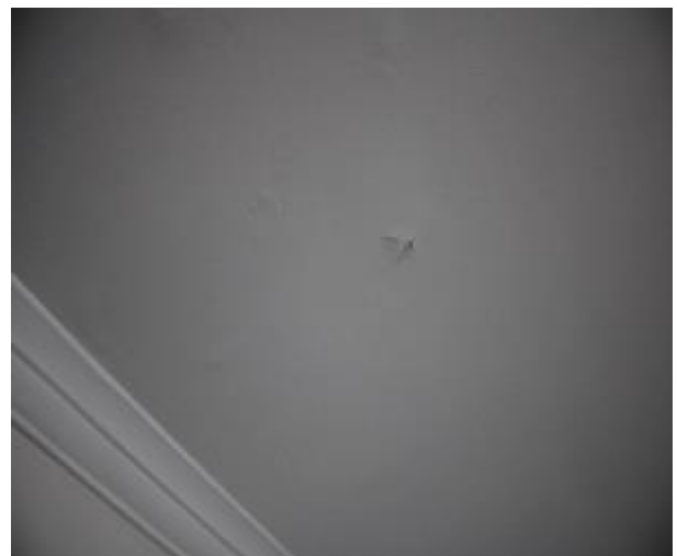
Figure 1618 - Paint flaking through bedroom 3 ceiling
