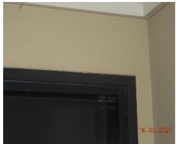
Figure 30 - Crack propagation through level 1 common area internal wall
