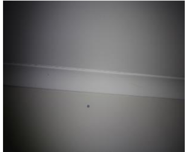
Figure 901 - Crack propagation through bedroom 2 ceiling
