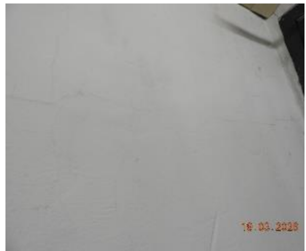
Figure 287 - Crack propagation through level 5 fire stairs internal wall
