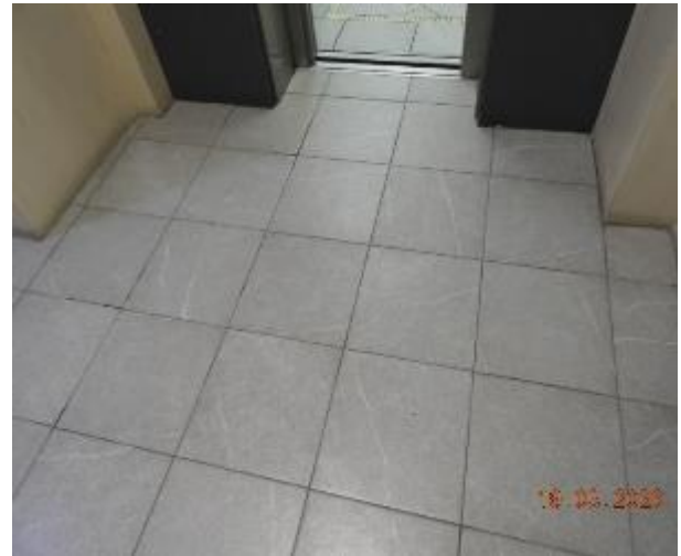
Figure 118 - General condition of level 4 common area floor tiles
