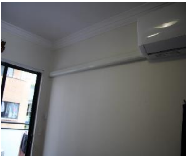
Figure 1107 - General condition of dining room internal wall
