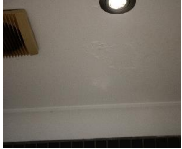
Figure 1057 - Paint flaking through ensuite bathroom ceiling
