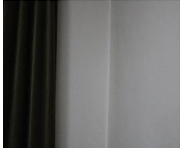
Figure 796 - Crack propagation through bedroom 1 internal wall
