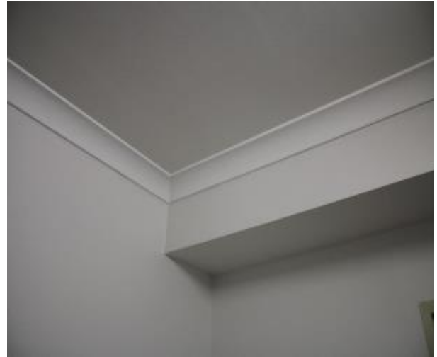
Figure 710 - General condition of dressing room ceiling
