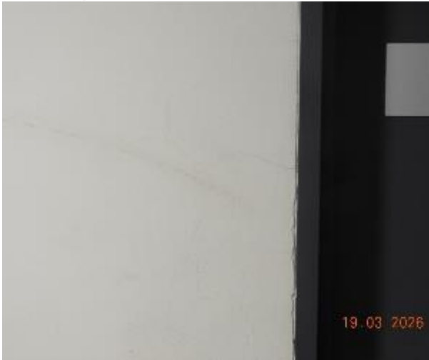
Figure 61 - Crack propagation through level 2 common area internal wall
