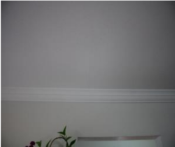
Figure 954 - Crack propagation through lounge room ceiling
