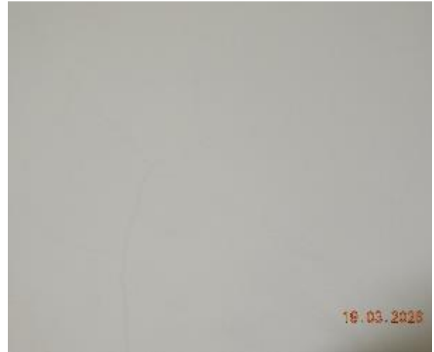
Figure 56 - Crack propagation through level 2 common area internal wall
