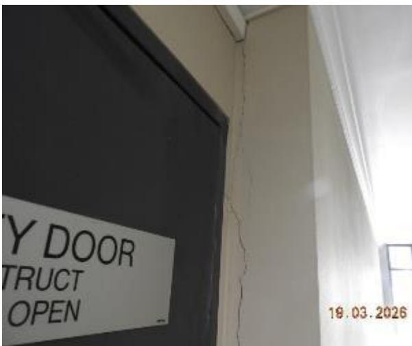
Figure 23 - Crack propagation through level 1 common area internal wall
