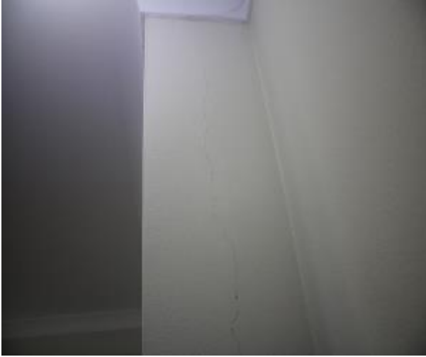
Figure 1199 - Crack propagation through bedroom 1 internal wall
