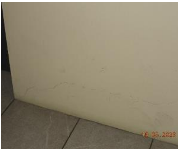
Figure 17 - Crack propagation through level 1 common area internal wall
