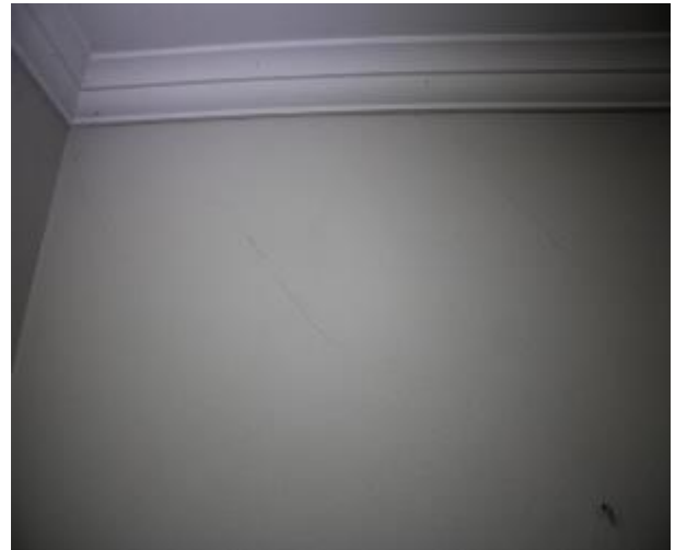
Figure 628 - Crack propagation through lounge room internal wall
