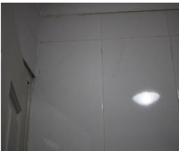
Figure 1221 - Crack propagation through ensuite bathroom internal wall
