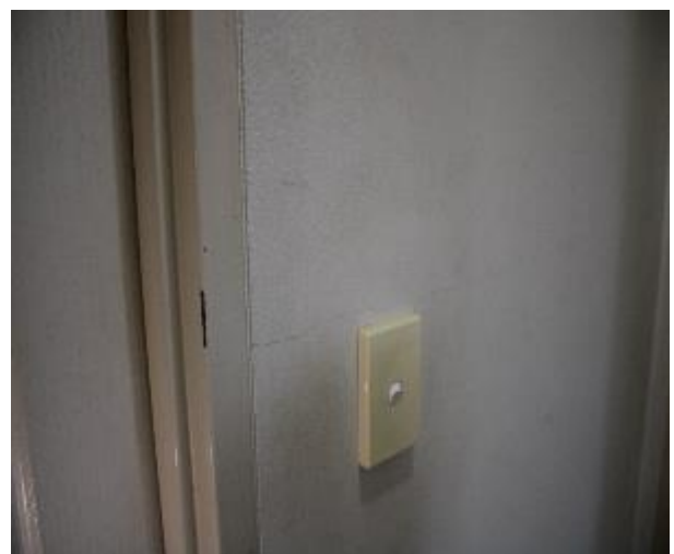
Figure 774 - Crack propagation through corridor internal wall
