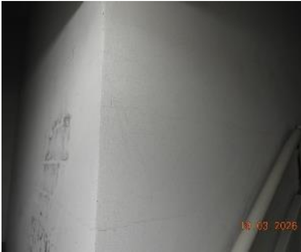
Figure 444 - Crack propagation through basement fire stairs internal wall
