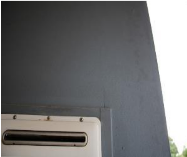
Figure 1086 - Crack propagation through external wall
