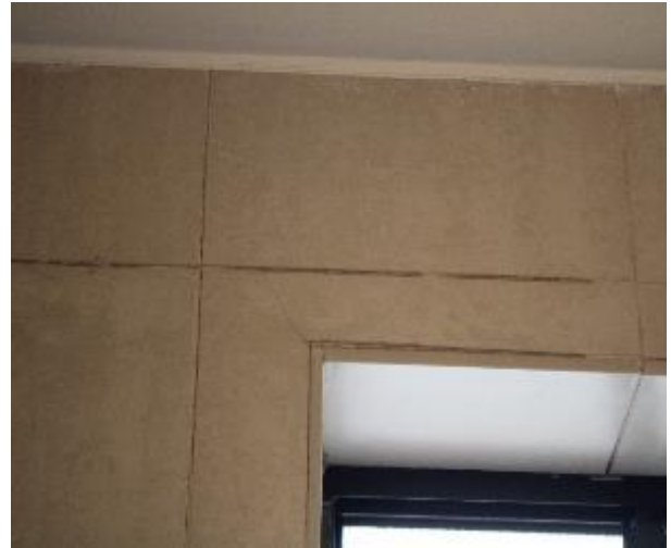
Figure 1590 - Crack propagation through bathroom 1 internal wall
