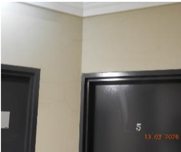
Figure 57 - Crack propagation through level 2 common area internal wall
