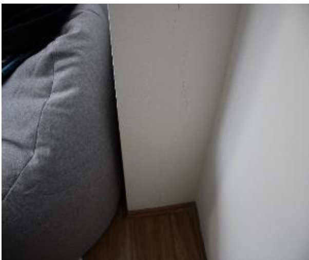
Figure 1197 - Crack propagation through bedroom 1 internal wall
