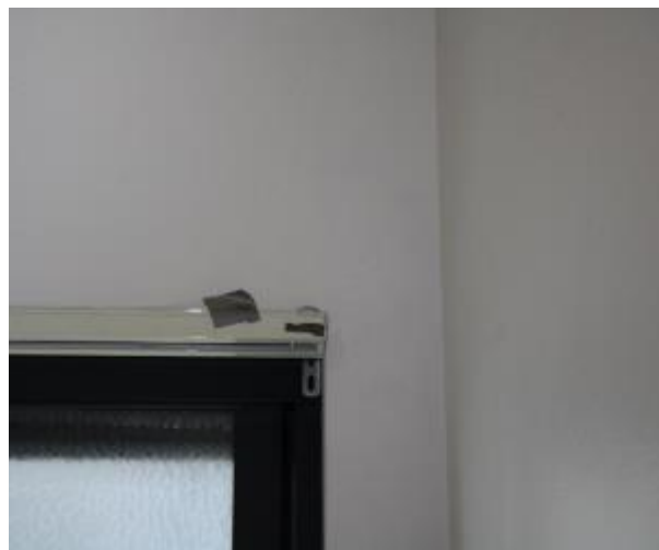
Figure 1548 - Crack propagation through bedroom 1 internal wall
