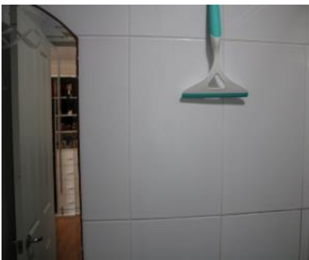
Figure 1215 - Crack propagation through ensuite bathroom internal wall
