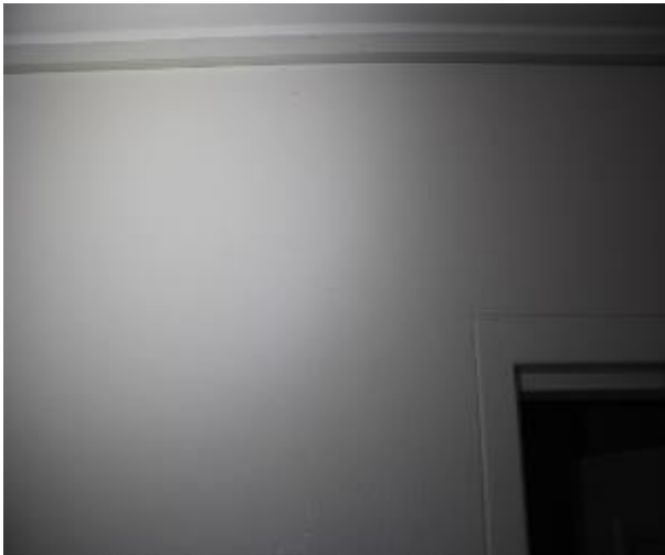
Figure 938 - Crack propagation through lounge room internal wall
