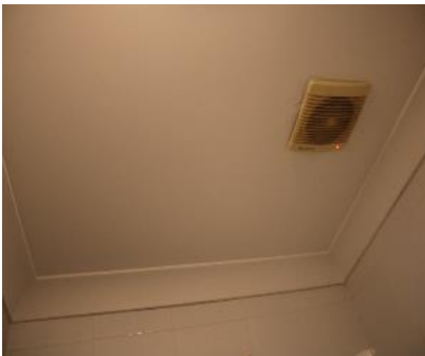
Figure 813 - General condition of ensuite bathroom ceiling
