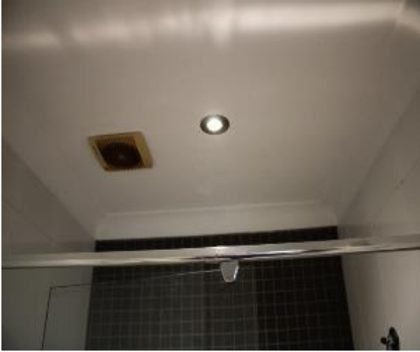
Figure 1056 - General condition of ensuite bathroom ceiling
