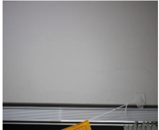
Figure 1069 - Crack propagation through bedroom 2 internal wall
