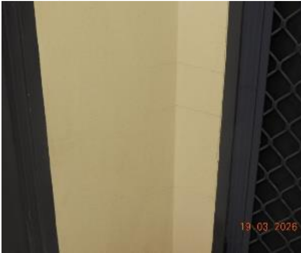
Figure 91 - Crack propagation through level 3 common area internal wall
