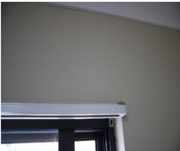
Figure 1414 - Crack propagation through study internal wall
