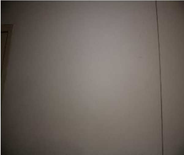
Figure 1276 - Crack propagation through lounge room internal wall
