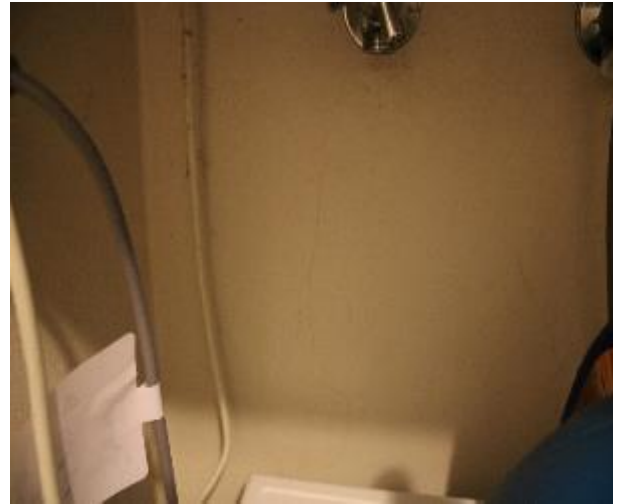
Figure 576 - Crack propagation through laundry internal wall
