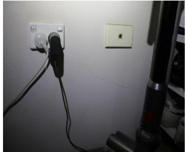
Figure 626 - Crack propagation through lounge room internal wall
