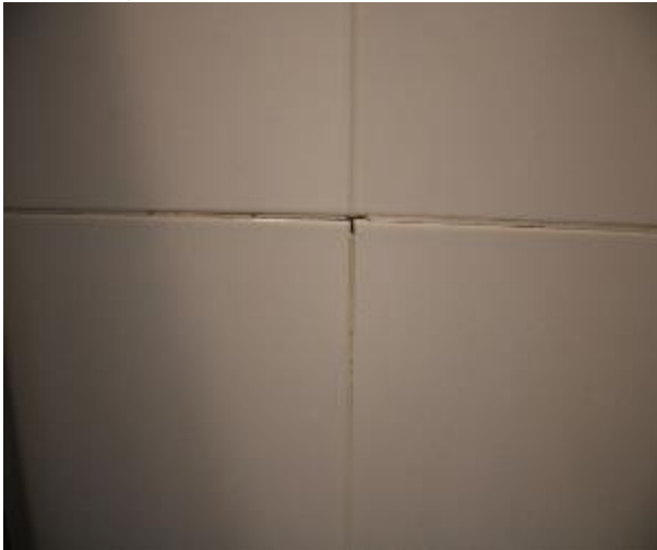
Figure 1625 - Crack propagation through ensuite bathroom internal wall
