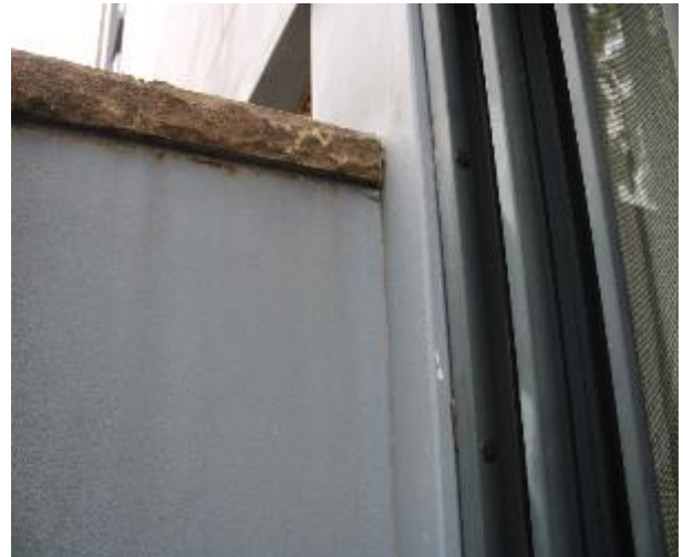
Figure 608 - Crack propagation through courtyard external wall
