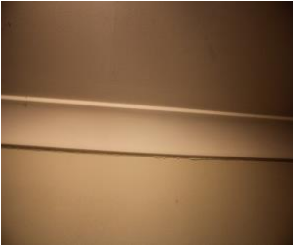
Figure 587 - Crack propagation through laundry ceiling
