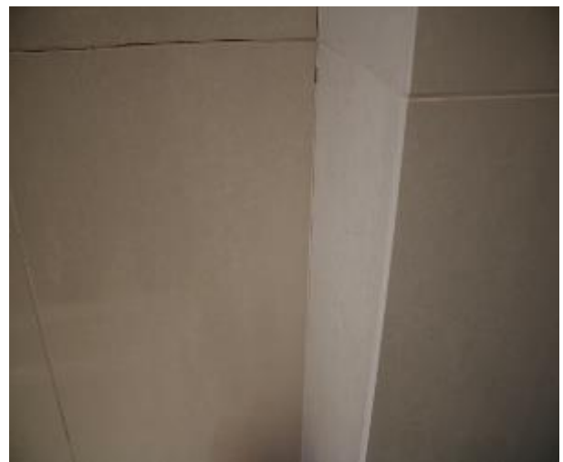
Figure 1013 - Crack propagation through bathroom 1 internal wall
