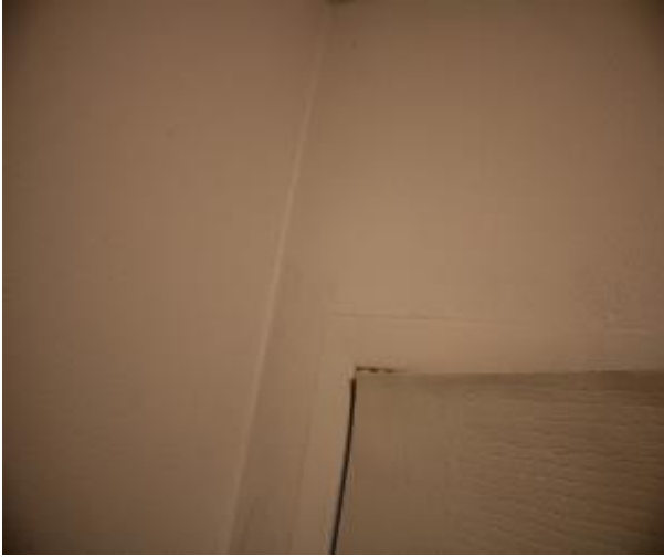
Figure 978 - Crack propagation through laundry internal wall
