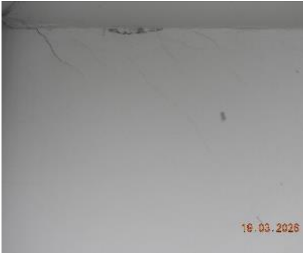
Figure 366 - Crack propagation through level 2 fire stairs internal wall
