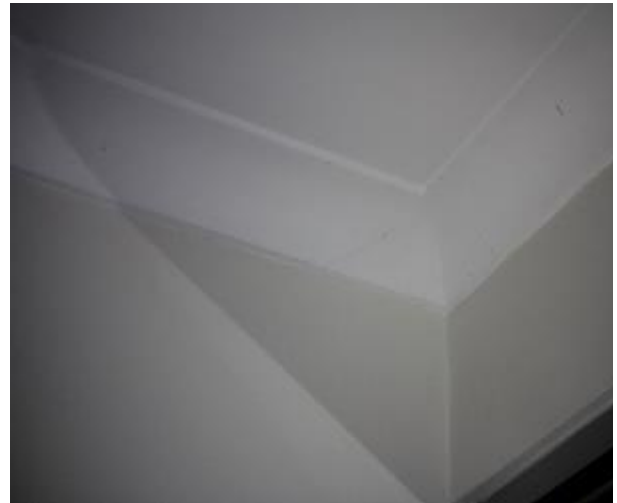
Figure 903 - Crack propagation through bedroom 2 ceiling
