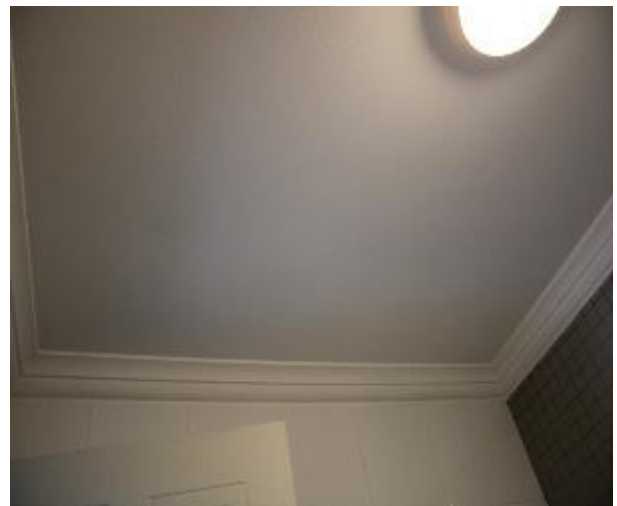
Figure 1634 - General condition of ensuite bathroom ceiling
