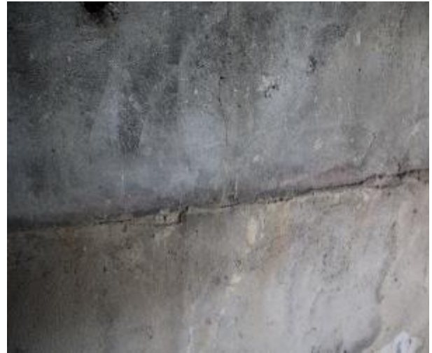
Figure 222 - Crack propagation through B1 fire stairs internal wall
