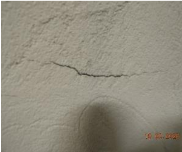
Figure 288 - Crack propagation through level 5 fire stairs internal wall
