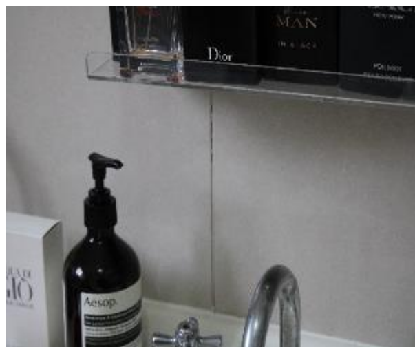
Figure 1178 - Crack propagation through bathroom 1 internal wall
