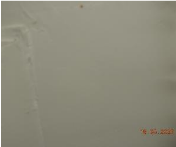
Figure 342 - Crack propagation through level 3 fire stairs underside stairs
