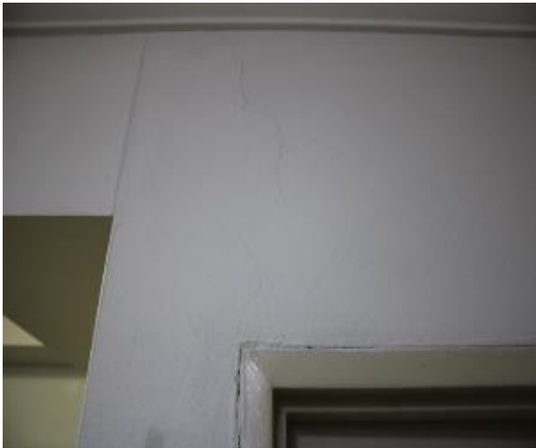
Figure 535 - Crack propagation through open kitchen/ lounge room internal wall
