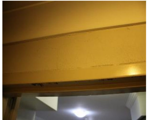
Figure 584 - Crack propagation through laundry internal wall
