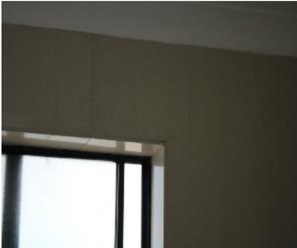
Figure 1163 - Crack propagation through bathroom 1 internal wall
