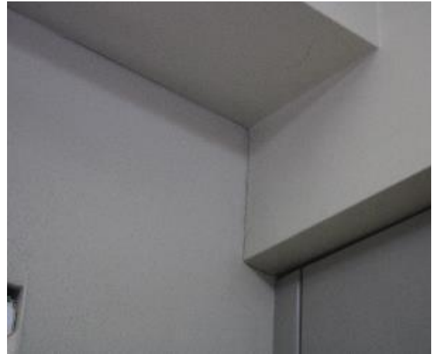
Figure 1311 - Crack propagation through kitchen internal wall
