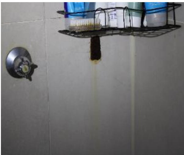
Figure 1173 - Crack propagation through bathroom 1 internal wall
