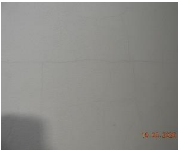
Figure 159 - Crack propagation through level 5 common area internal wall
