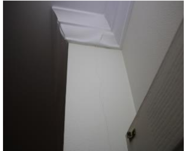
Figure 1146 - Crack propagation through dining room internal wall
