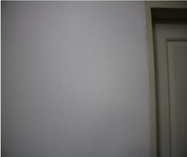
Figure 789 - Crack propagation through bedroom 1 internal wall
