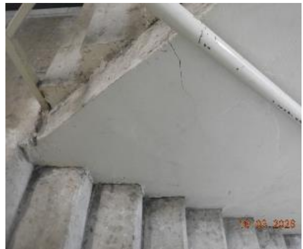
Figure 399 - Crack propagation through level 1 fire stairs internal wall
