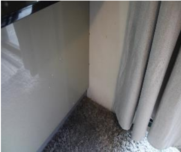
Figure 745 - Crack propagation through open kitchen/ lounge room internal wall
