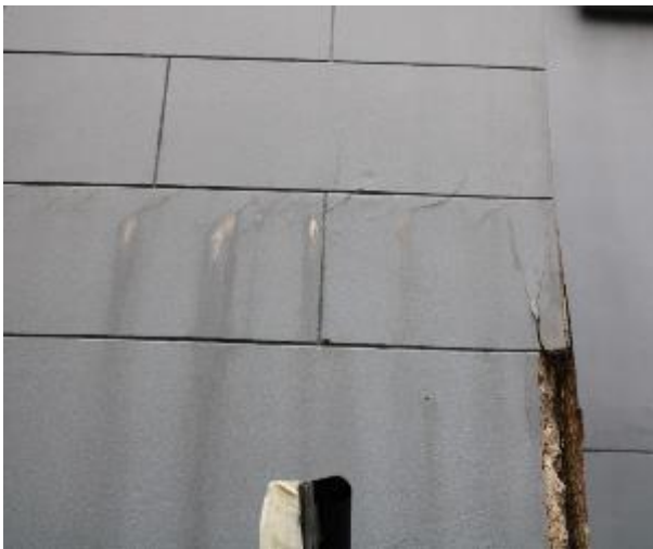
Figure 601 - Crack propagation through external wall
