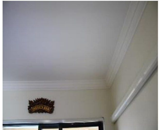
Figure 1118 - General condition of dining room ceiling
