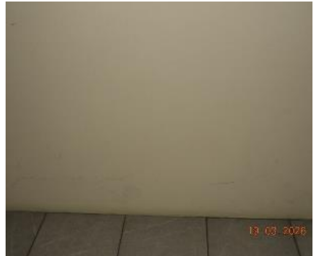
Figure 16 - Crack propagation through level 1 common area internal wall
