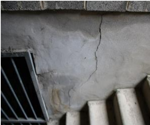
Figure 259 - Crack propagation through level 1 fire stairs internal wall
