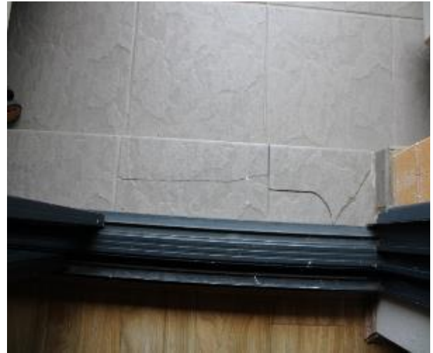
Figure 1248 - Crack propagation through balcony floor tiles
