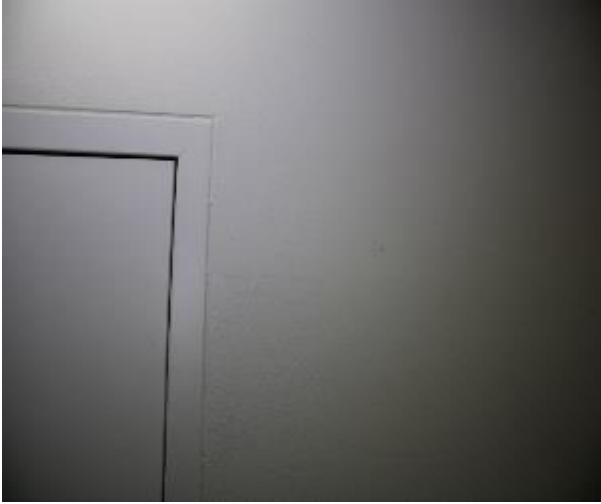
Figure 948 - Crack propagation through lounge room internal wall
