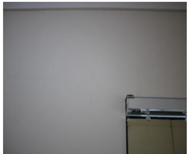
Figure 1232 - Crack propagation through bedroom 2 internal wall
