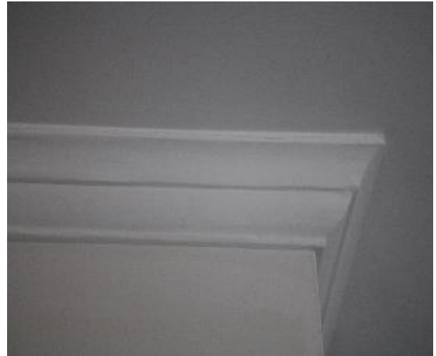
Figure 1476 - Crack propagation through open kitchen/ lounge room ceiling
