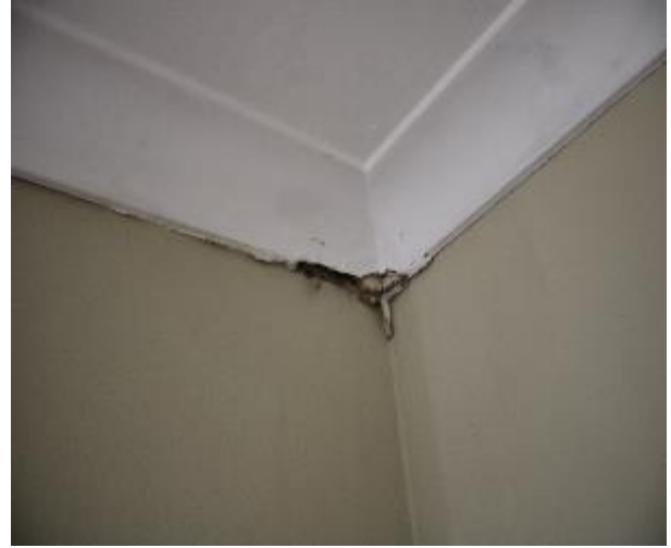
Figure 1389 - Water damage evident through bedroom 1 ceiling
