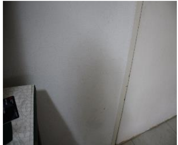
Figure 730 - Crack propagation through open kitchen/ lounge room internal wall
