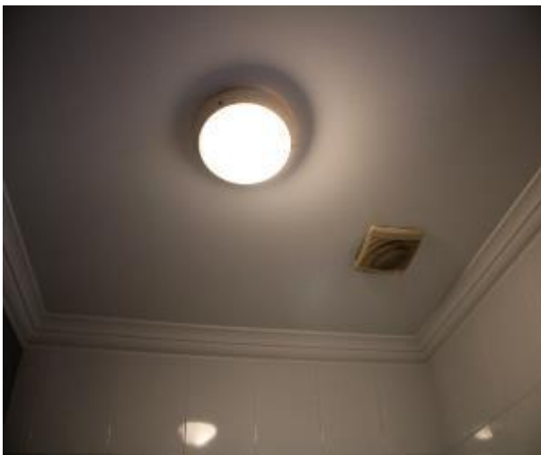
Figure 1633 - General condition of ensuite bathroom ceiling
