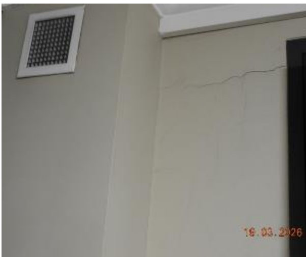
Figure 179 - Crack propagation through level 5 common area internal wall
