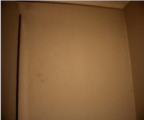
Figure 581 - Crack propagation through laundry internal wall
