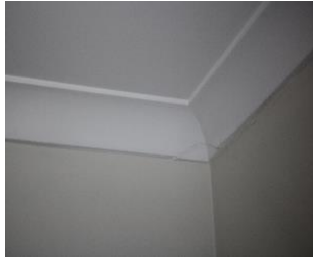
Figure 1244 - Crack propagation through bedroom 2 ceiling
