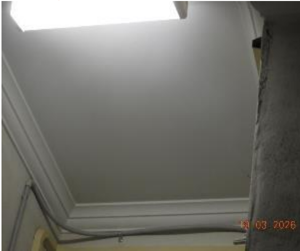
Figure 312 - General condition of level 5 fire stairs ceiling
