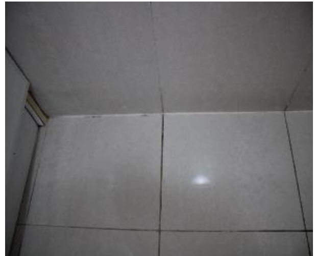
Figure 694 - Crack propagation through bathroom 1 floor tiles
