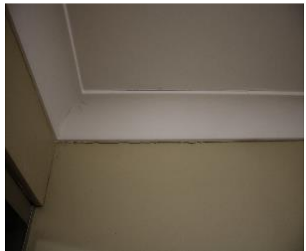
Figure 1393 - Crack propagation through bedroom 1 ceiling
