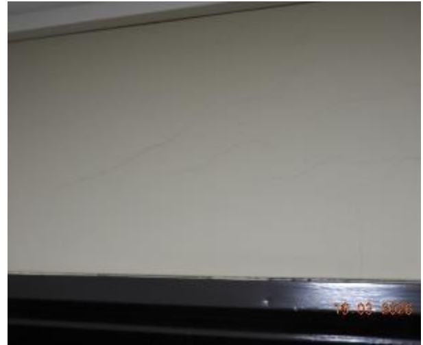
Figure 68 - Crack propagation through level 2 common area internal wall
