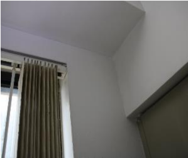
Figure 1469 - Crack propagation through open kitchen/ lounge room internal wall
