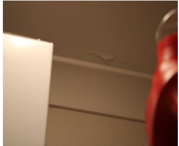
Figure 1140 - Crack propagation through laundry ceiling
