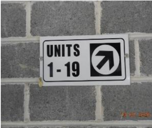
Figure 276 - The following images display the condition of the fire stairs from Level 5 to B2
