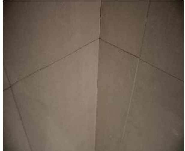
Figure 1005 - Crack propagation through bathroom 1 internal wall
