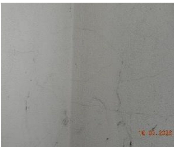
Figure 454 - Crack propagation through basement fire stairs internal wall
