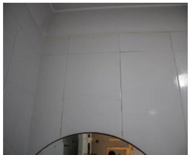
Figure 1216 - Crack propagation through ensuite bathroom internal wall
