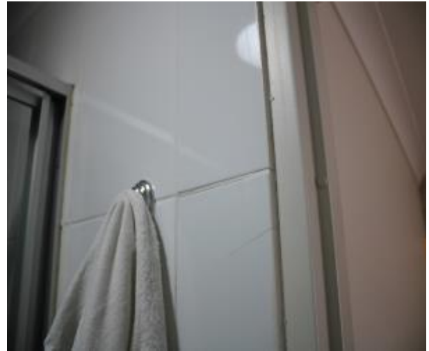
Figure 1224 - Crack propagation through ensuite bathroom internal wall
