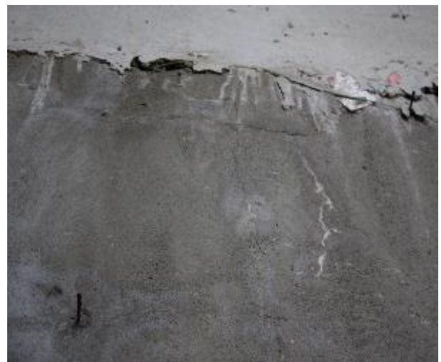
Figure 226 - Crack propagation through B1 fire stairs internal wall
