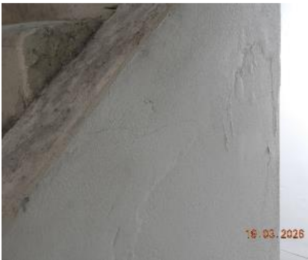
Figure 398 - Crack propagation through level 1 fire stairs internal wall
