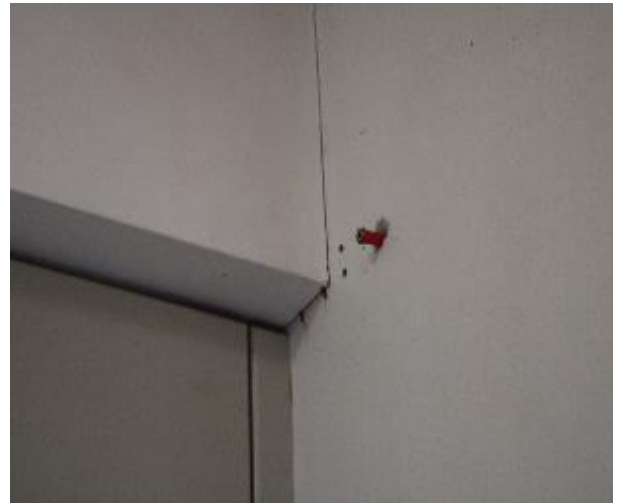
Figure 754 - Crack propagation through open kitchen/ lounge room internal wall
