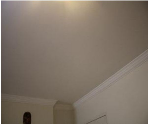
Figure 1115 - General condition of dining room ceiling
