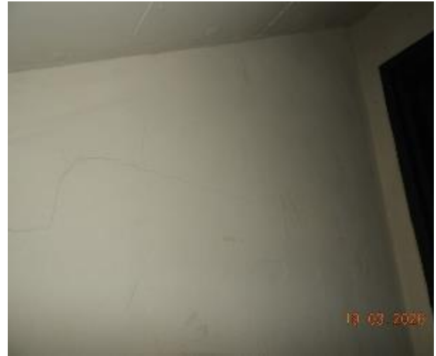
Figure 445 - Crack propagation through basement fire stairs internal wall
