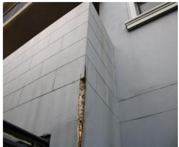
Figure 598 - Water damage evident through external wall
