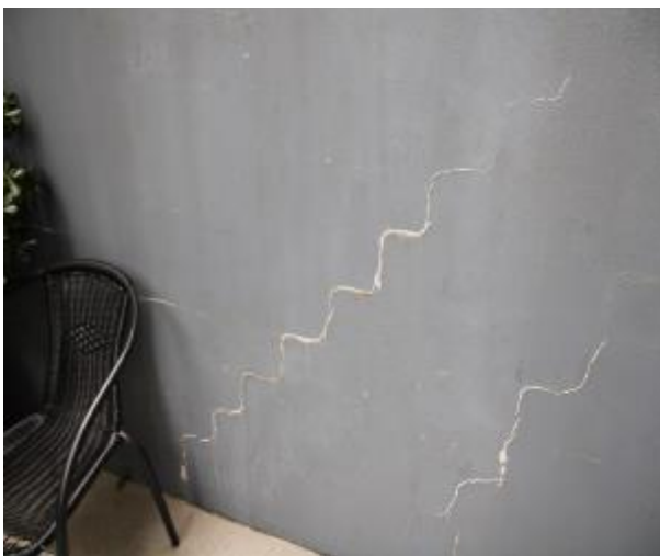
Figure 609 - Crack propagation through courtyard external wall
