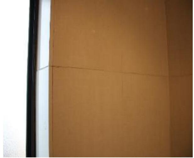
Figure 1003 - Crack propagation through bathroom 1 internal wall
