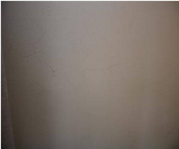
Figure 741 - Crack propagation through open kitchen/ lounge room internal wall
