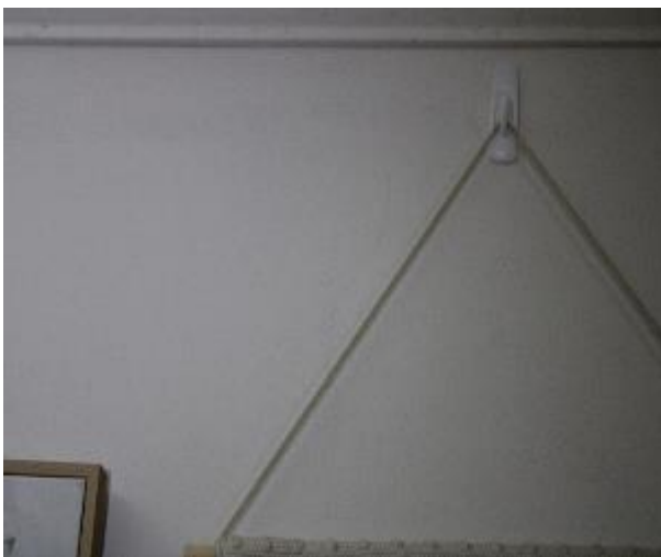
Figure 531 - Crack propagation through open kitchen/ lounge room internal wall
