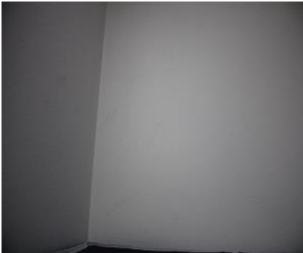
Figure 541 - Crack propagation through open kitchen/ lounge room internal wall
