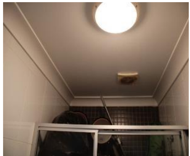
Figure 911 - General condition of ensuite bathroom ceiling
