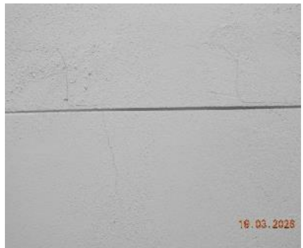
Figure 413 - Crack propagation through level 1 fire stairs underside stairs
