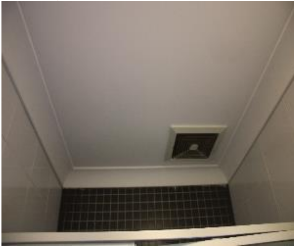
Figure 1412 - General condition of ensuite bathroom ceiling
