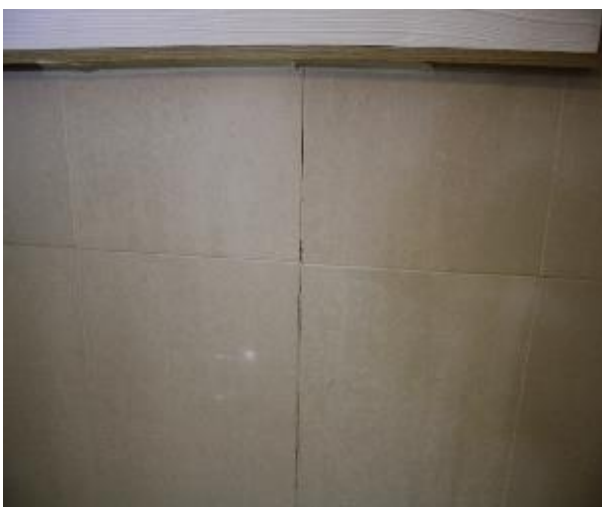
Figure 561 - Crack propagation through bathroom 1 internal wall
