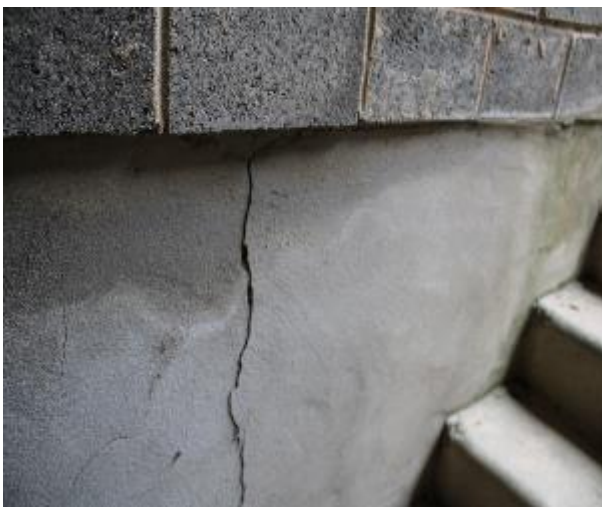
Figure 261 - Crack propagation through level 1 fire stairs internal wall
