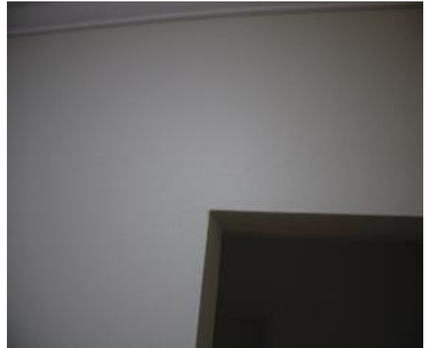
Figure 1104 - Crack propagation through dining room internal wall
