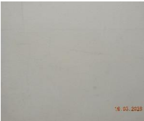
Figure 153 - Crack propagation through level 5 common area internal wall
