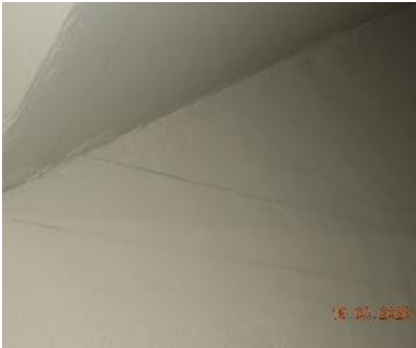
Figure 350 - Crack propagation through level 3 fire stairs internal wall
