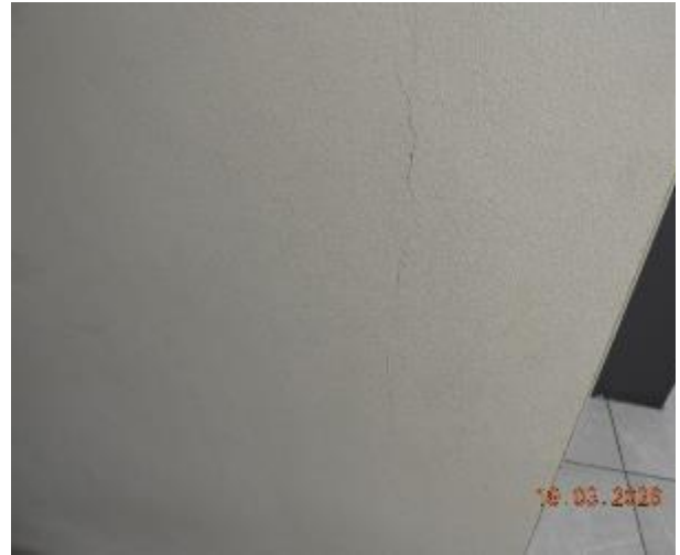
Figure 50 - Crack propagation through level 2 common area internal wall
