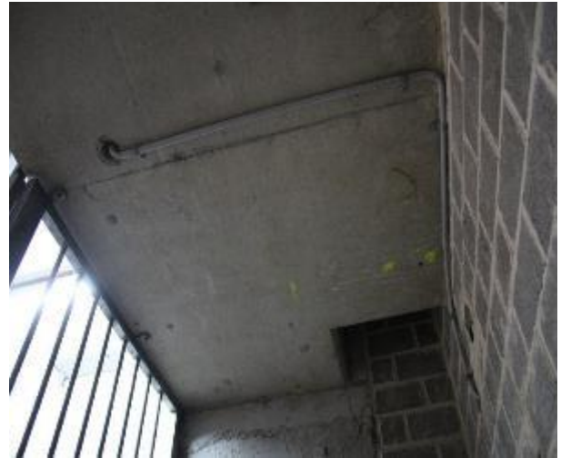
Figure 234 - General condition of B1 fire stairs underside slab
