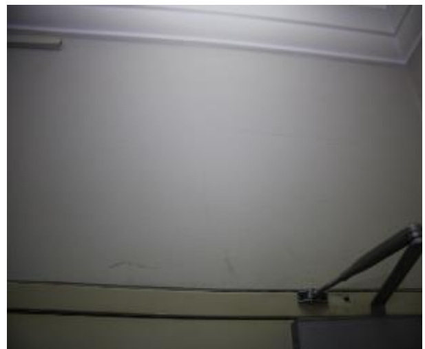
Figure 732 - Crack propagation through open kitchen/ lounge room internal wall
