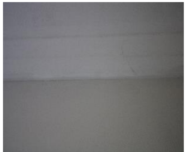
Figure 1558 - Crack propagation through bedroom 1 ceiling
