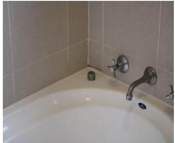
Figure 1349 - Crack propagation through bathroom 1 internal wall
