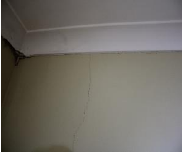
Figure 1382 - Crack propagation through bedroom 1 internal wall
