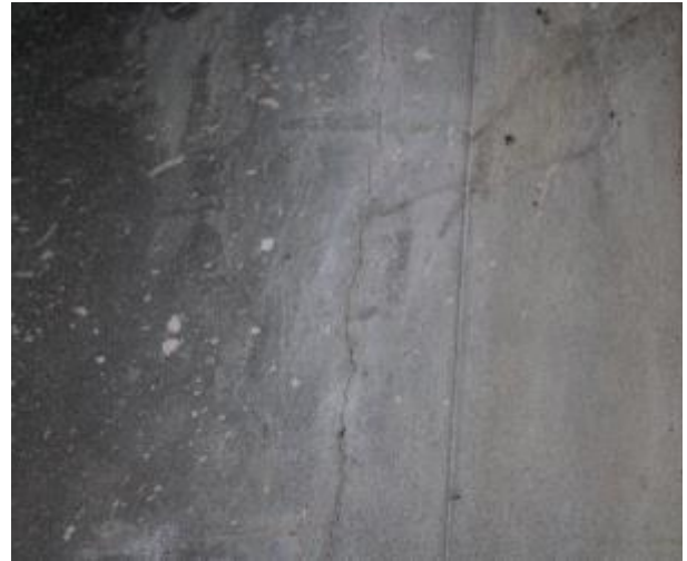
Figure 204 - Crack propagation through B2 fire stairs internal wall
