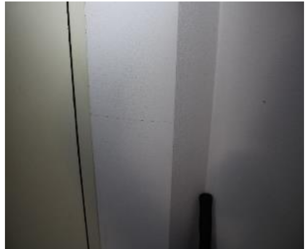
Figure 622 - Crack propagation through lounge room internal wall
