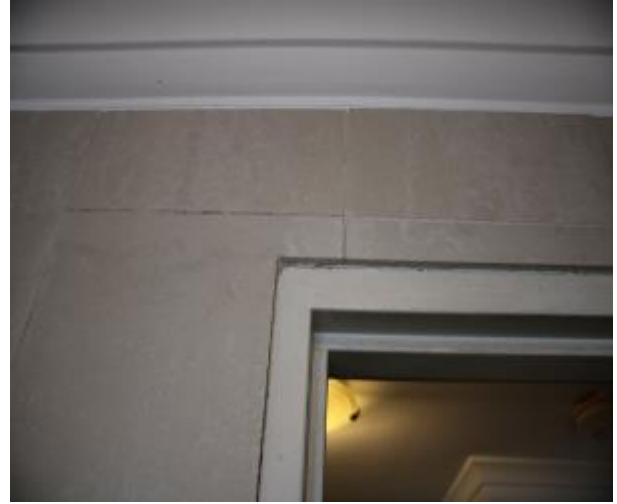
Figure 1596 - Crack propagation through bathroom 1 internal wall
