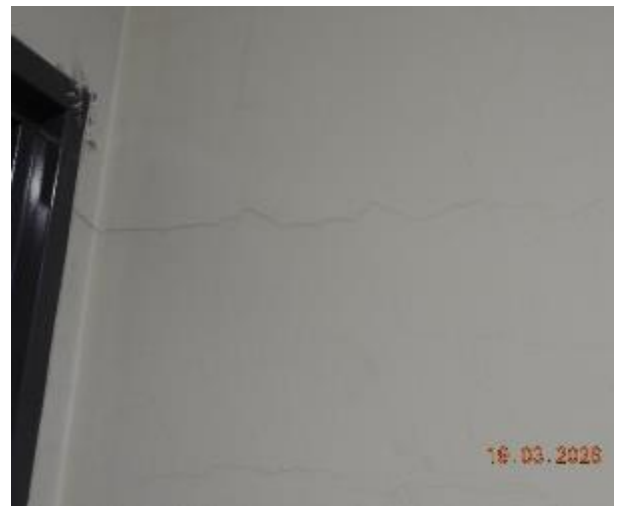
Figure 136 - Crack propagation through level 4 common area internal wall
