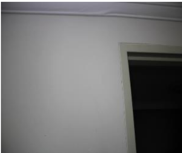
Figure 1609 - Crack propagation through bedroom 3 internal wall
