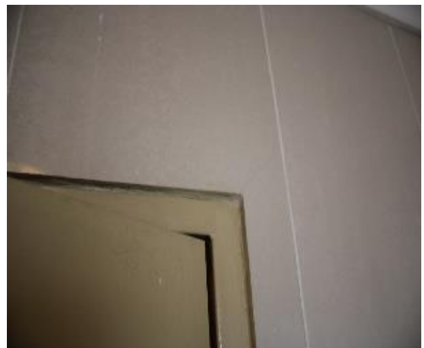
Figure 1357 - Crack propagation through bathroom 1 internal wall
