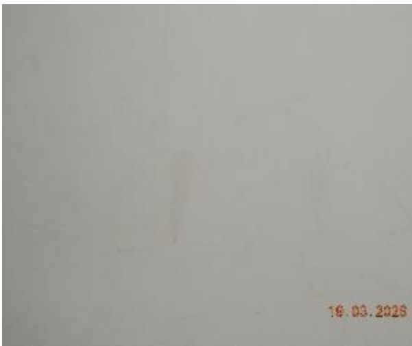
Figure 63 - Crack propagation through level 2 common area internal wall
