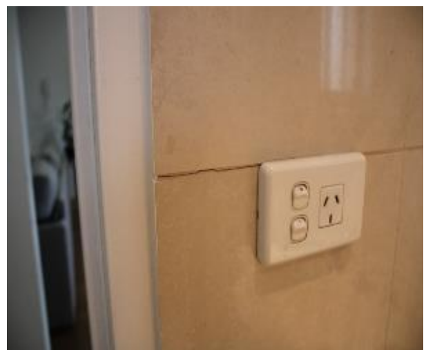
Figure 1019 - Crack propagation through bathroom 1 internal wall
