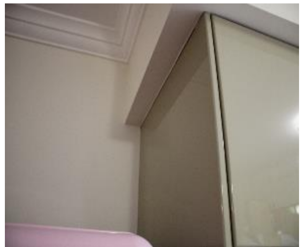
Figure 1126 - Crack propagation through kitchen internal wall
