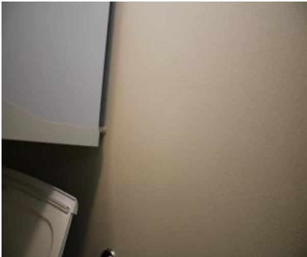
Figure 1318 - Crack propagation through laundry internal wall
