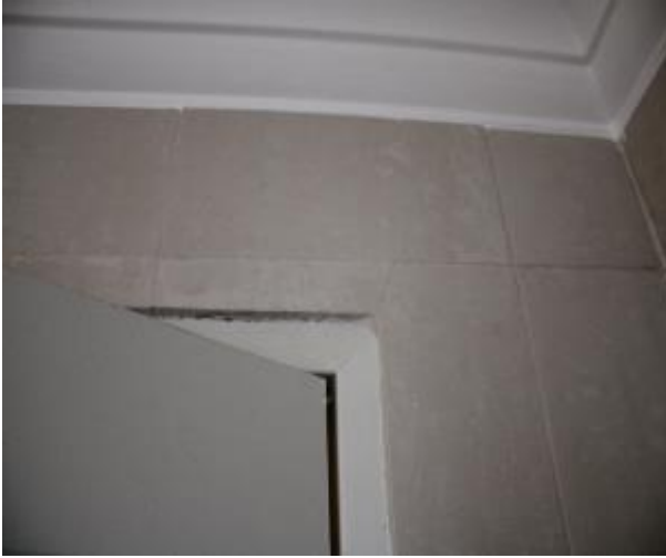
Figure 1595 - Crack propagation through bathroom 1 internal wall
