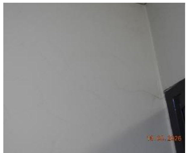
Figure 126 - Crack propagation through level 4 common area internal wall
