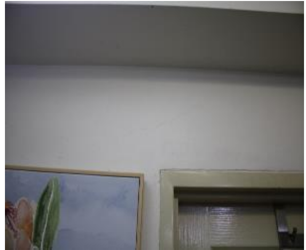
Figure 534 - Crack propagation through open kitchen/ lounge room internal wall
