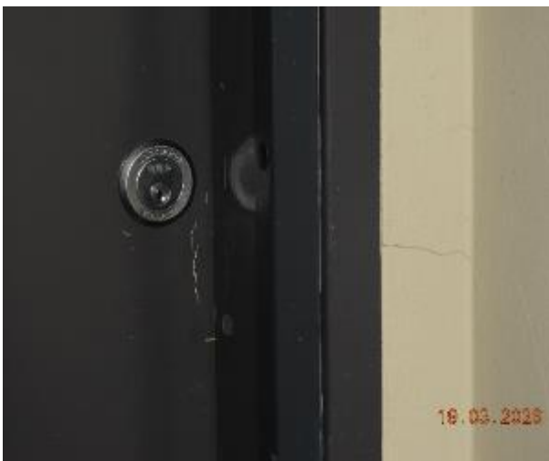
Figure 29 - Crack propagation through level 1 common area internal wall
