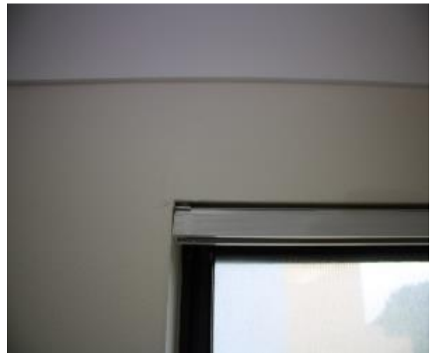
Figure 1186 - Crack propagation through bedroom 1 internal wall
