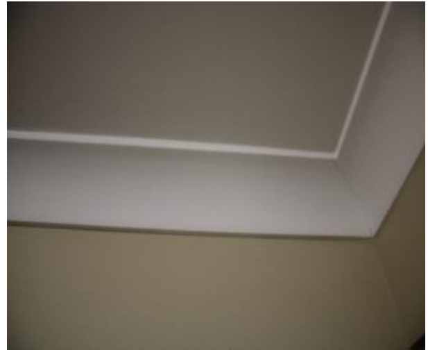
Figure 1395 - Crack propagation through bedroom 1 ceiling
