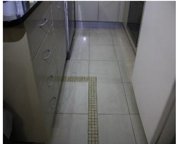
Figure 474 - General condition of open kitchen/ lounge room floor tiles
