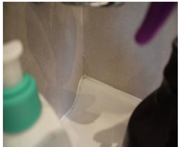
Figure 1023 - Crack propagation through bathroom 1 internal wall
