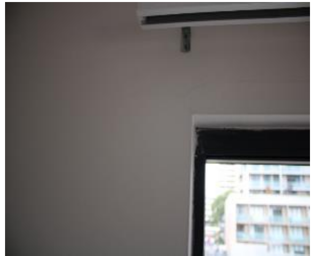
Figure 1059 - Crack propagation through bedroom 2 internal wall
