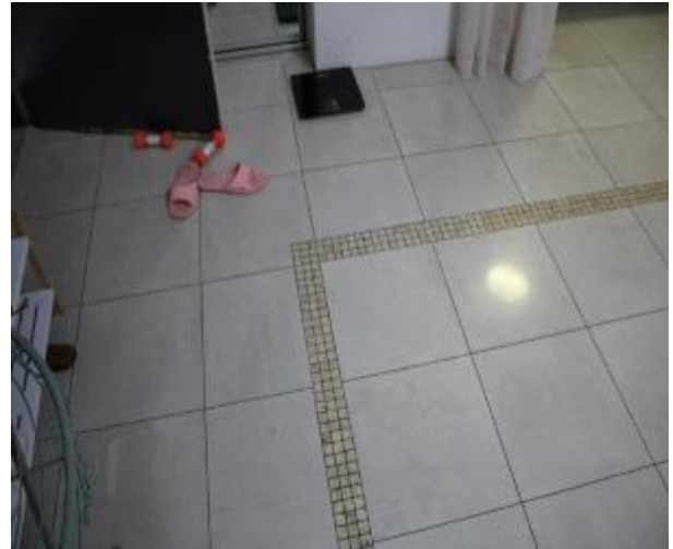
Figure 522 - General condition of open kitchen/ lounge room floor tiles
