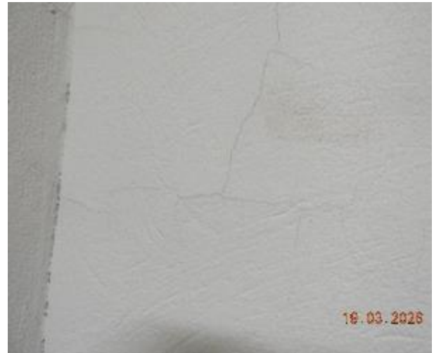
Figure 285 - Crack propagation through level 5 fire stairs internal wall
