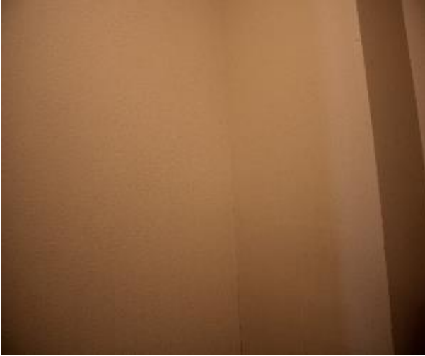
Figure 1322 - Crack propagation through laundry internal wall
