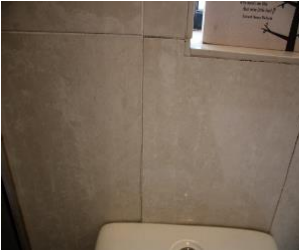
Figure 1589 - Crack propagation through bathroom 1 internal wall
