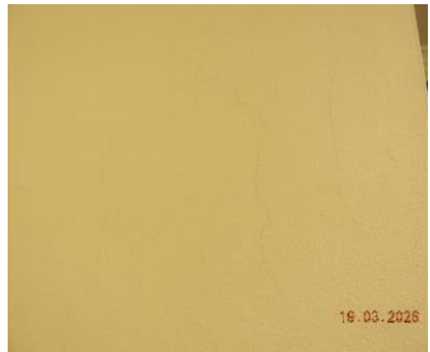
Figure 82 - Crack propagation through level 3 common area internal wall
