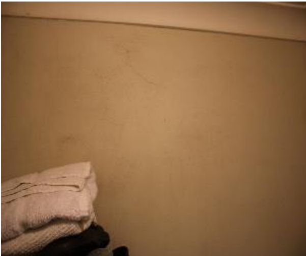
Figure 571 - Crack propagation through laundry internal wall
