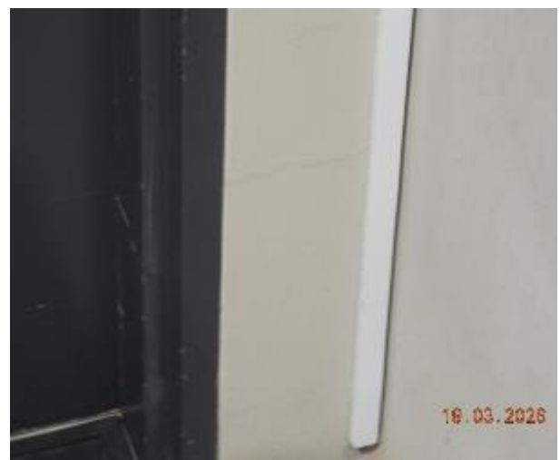
Figure 174 - Crack propagation through level 5 common area internal wall
