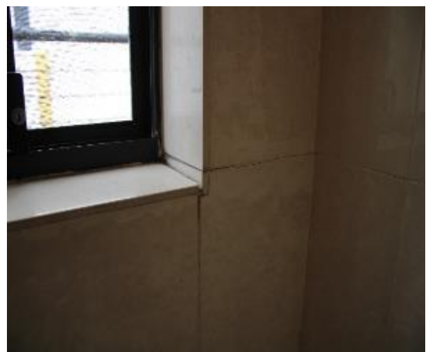
Figure 1588 - Crack propagation through bathroom 1 internal wall
