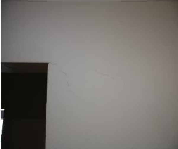
Figure 1288 - Crack propagation through lounge room internal wall
