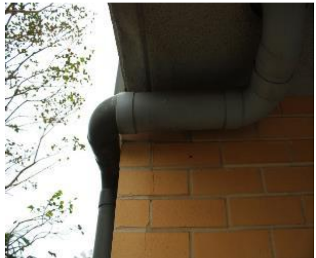
Figure 840 - Crack propagation through external wall
