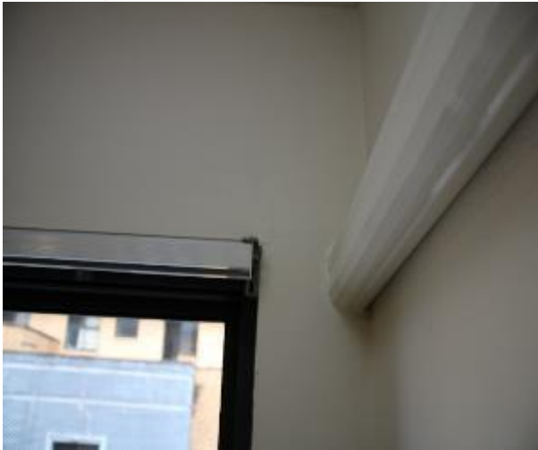
Figure 1109 - Crack propagation through dining room internal wall
