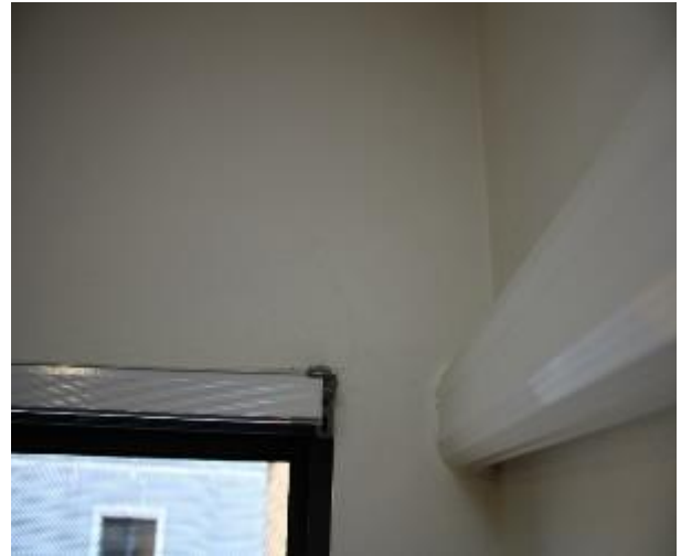
Figure 1110 - Crack propagation through dining room internal wall
