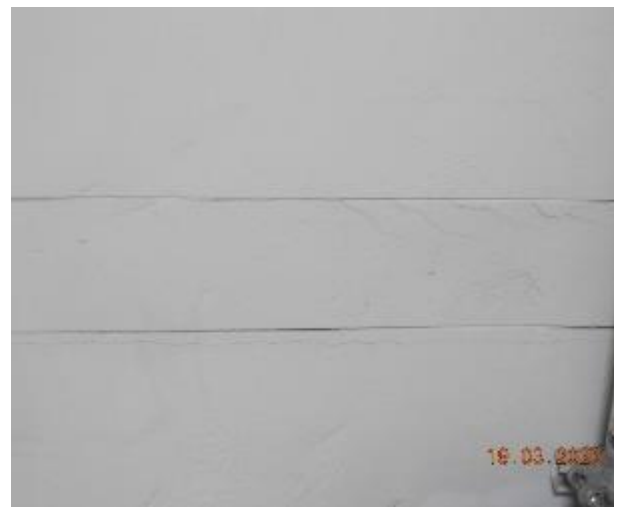
Figure 335 - Crack propagation through level 3 fire stairs internal wall
