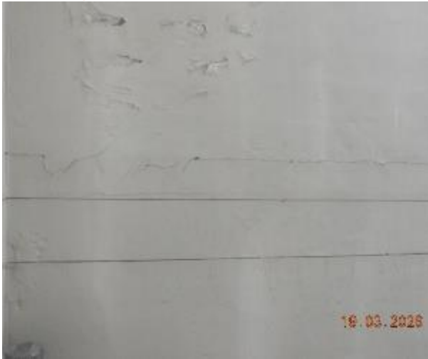
Figure 294 - Crack propagation and paint flaking through level 5 fire stairs internal wall
