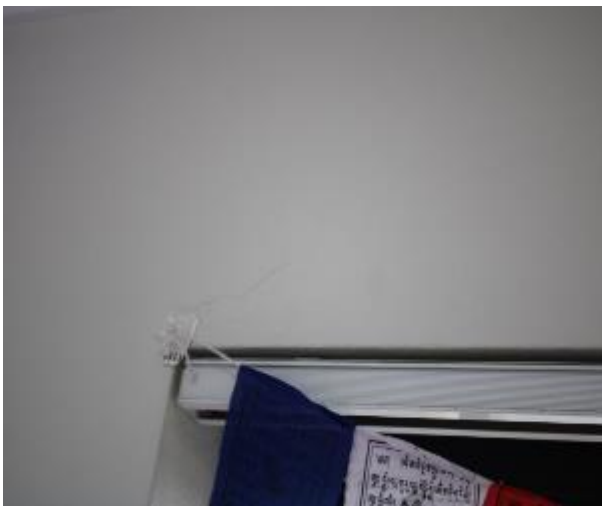
Figure 1070 - Crack propagation through bedroom 2 internal wall
