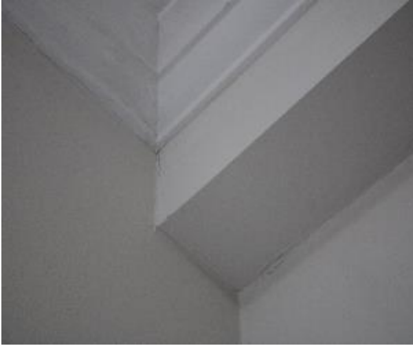
Figure 1553 - Crack propagation through bedroom 1 internal wall
