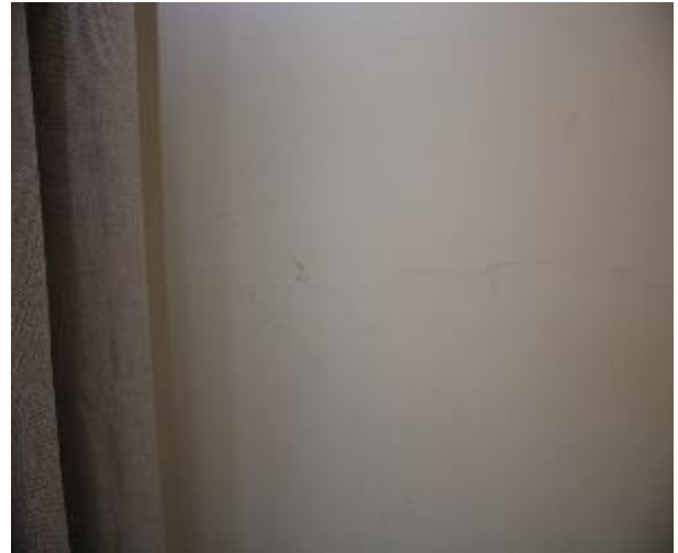
Figure 740 - Crack propagation through open kitchen/ lounge room internal wall
