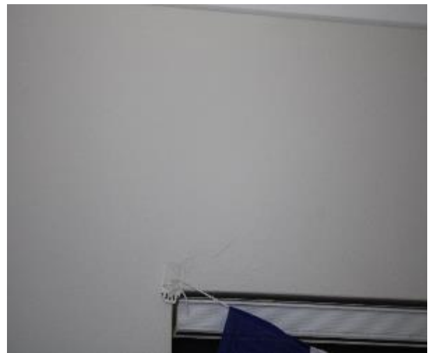
Figure 1071 - Crack propagation through bedroom 2 internal wall
