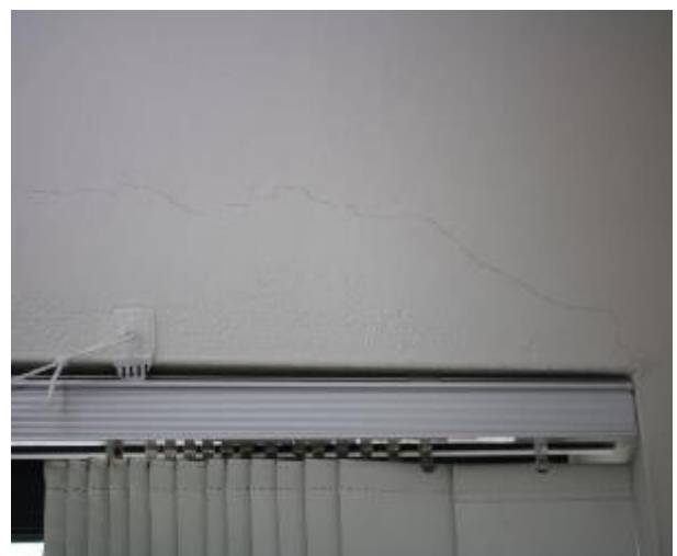
Figure 1067 - Crack propagation through bedroom 2 internal wall
