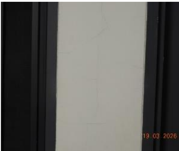
Figure 177 - Crack propagation through level 5 common area internal wall
