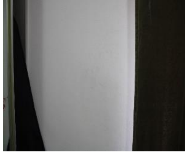
Figure 794 - Crack propagation through bedroom 1 internal wall
