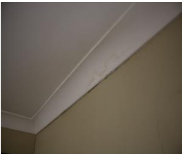
Figure 1392 - Crack propagation through bedroom 1 ceiling
