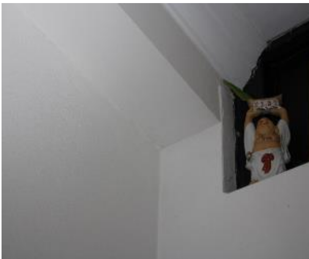
Figure 1561 - Crack propagation through bedroom 1 ceiling
