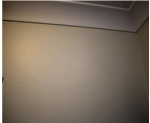
Figure 1152 - Crack propagation through corridor internal wall
