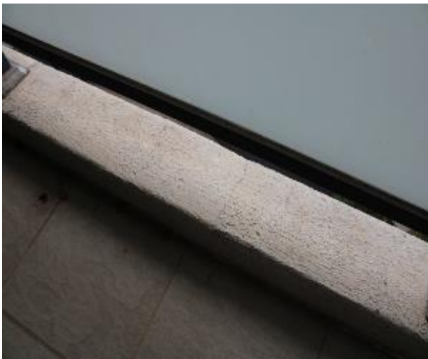
Figure 831 - Crack propagation through external wall
