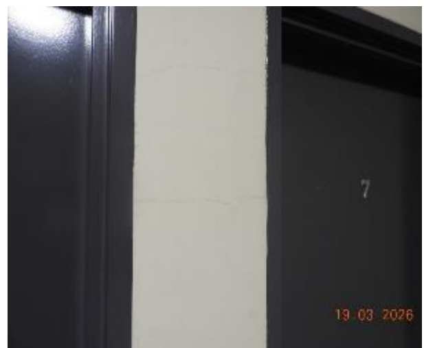
Figure 66 - Crack propagation through level 2 common area internal wall
