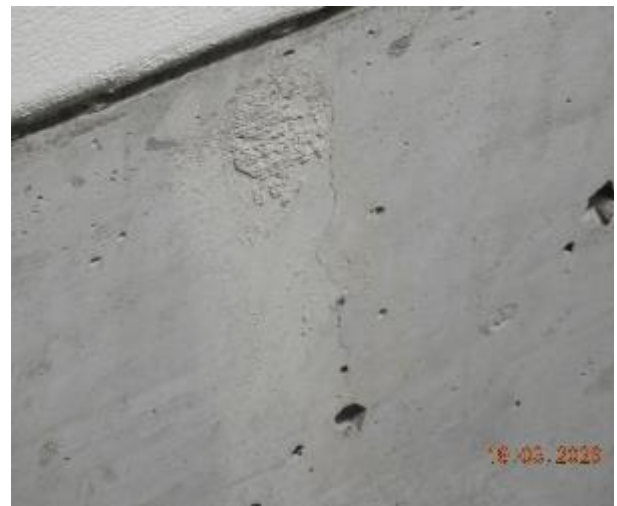
Figure 453 - Crack propagation through basement fire stairs internal wall
