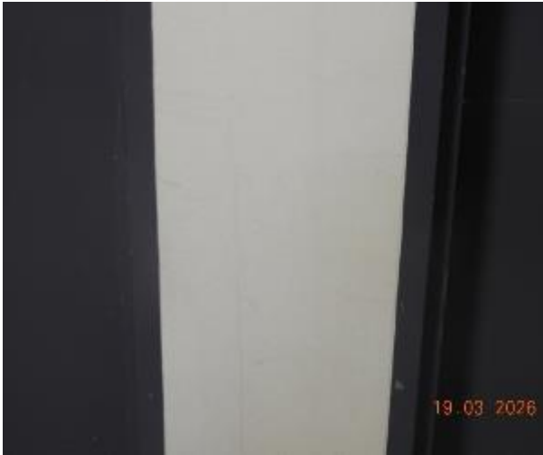
Figure 139 - Crack propagation through level 4 common area internal wall
