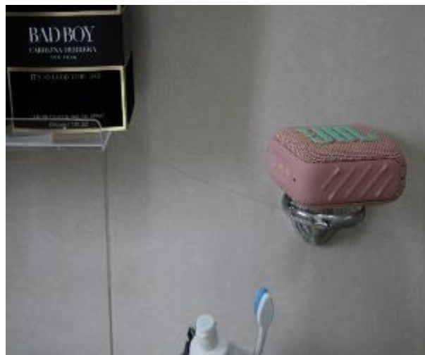
Figure 1176 - Crack propagation through bathroom 1 internal wall
