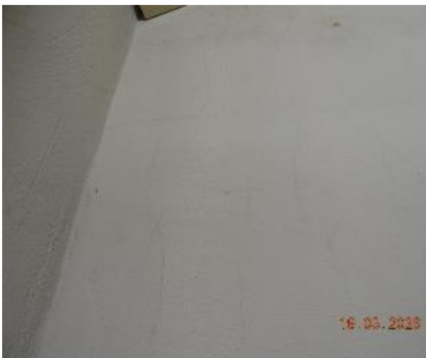
Figure 286 - Crack propagation through level 5 fire stairs internal wall
