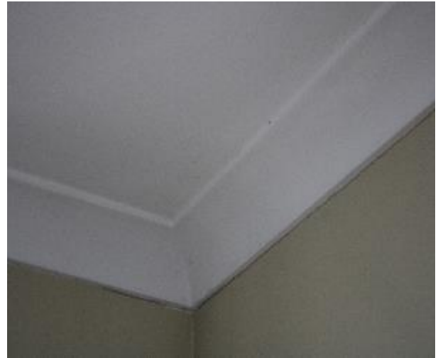
Figure 1431 - Crack propagation through study ceiling
