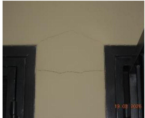
Figure 28 - Crack propagation through level 1 common area internal wall
