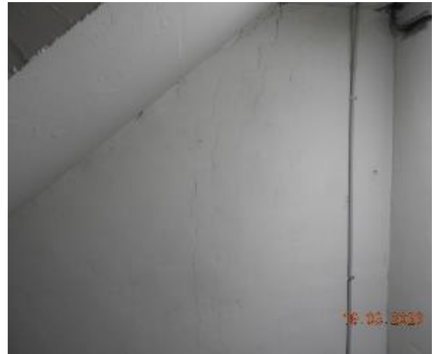
Figure 321 - Crack propagation through level 4 fire stairs internal wall
