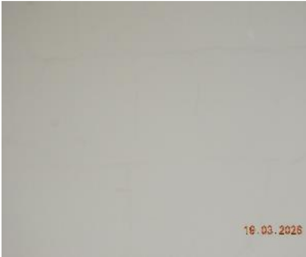
Figure 169 - Crack propagation through level 5 common area internal wall
