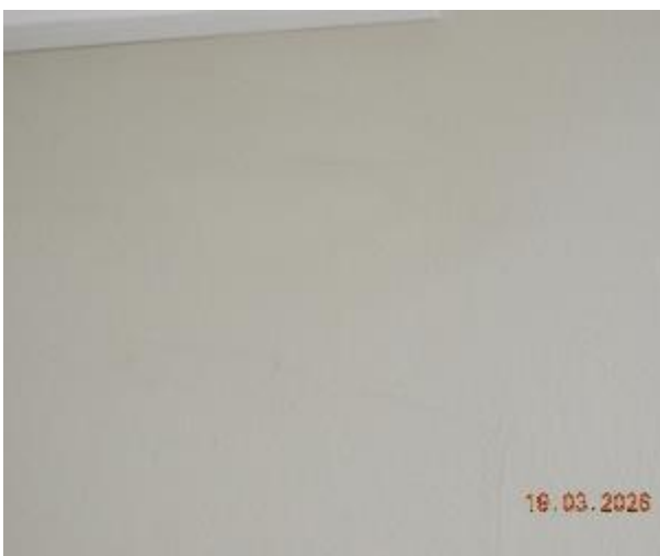
Figure 53 - Crack propagation through level 2 common area internal wall
