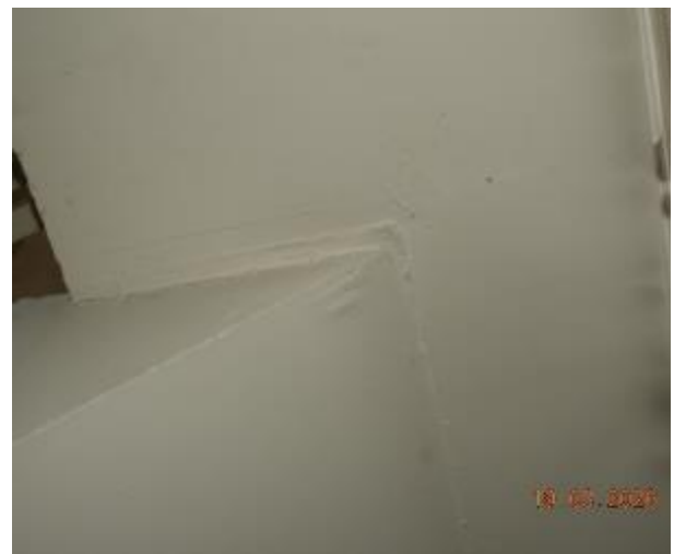
Figure 341 - Crack propagation through level 3 fire stairs underside stairs
