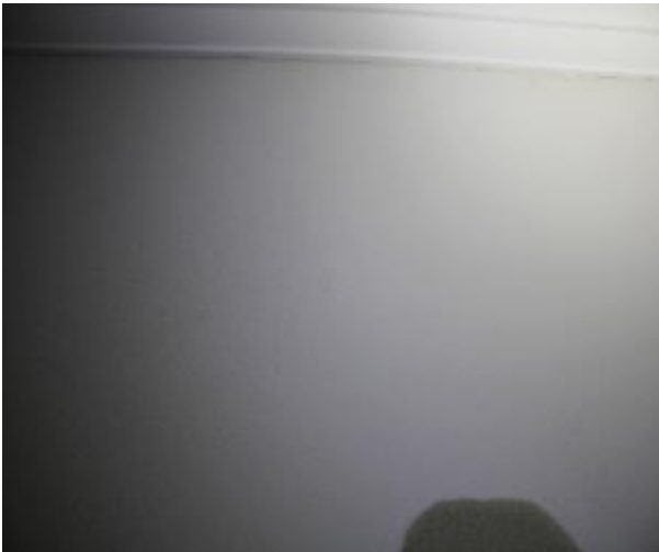
Figure 627 - Crack propagation through lounge room internal wall
