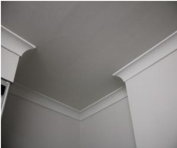
Figure 711 - General condition of dressing room ceiling
