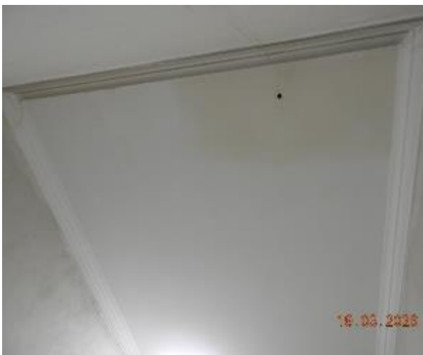
Figure 310 - General condition of level 5 fire stairs ceiling
