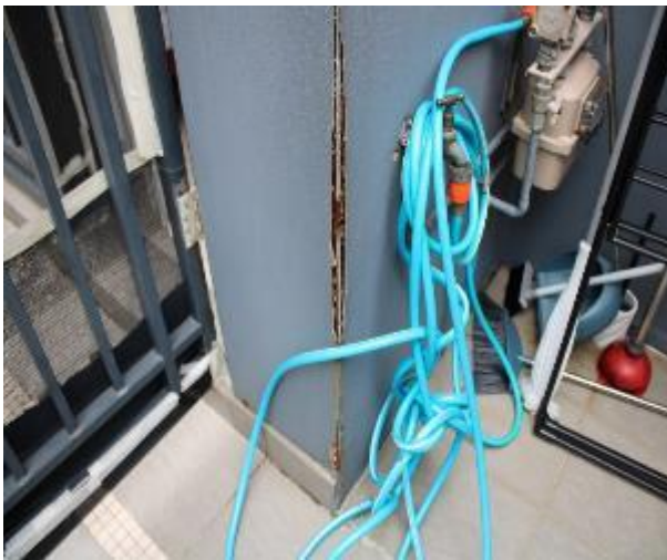
Figure 595 - Water damage evident through external wall
