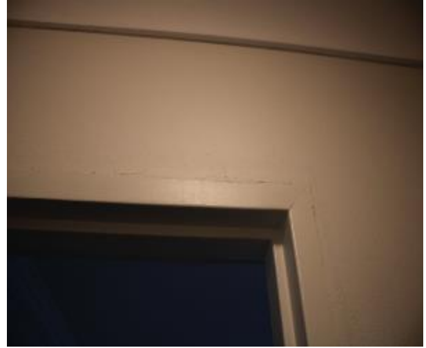
Figure 979 - Crack propagation through laundry internal wall
