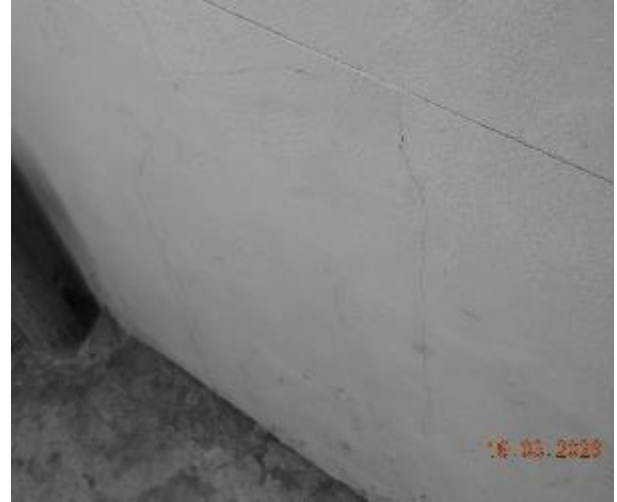
Figure 403 - Crack propagation through level 1 fire stairs internal wall
