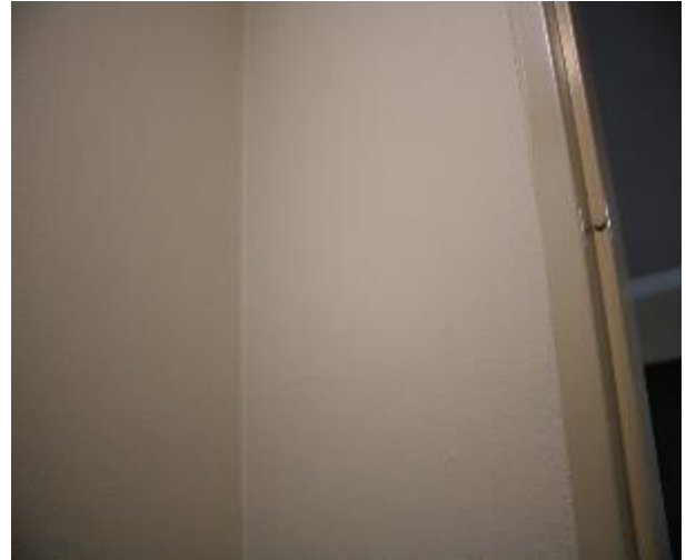
Figure 1325 - Crack propagation through laundry internal wall
