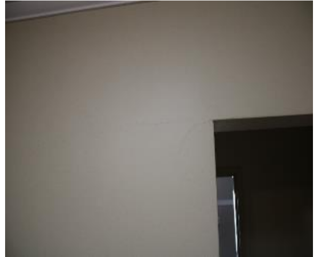
Figure 1289 - Crack propagation through lounge room internal wall
