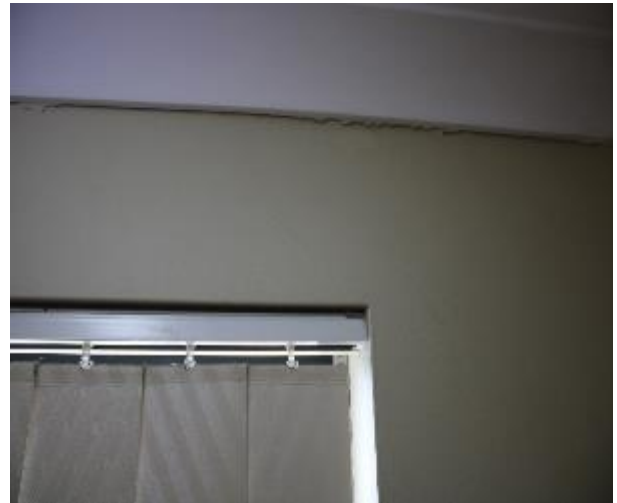
Figure 1367 - Crack propagation through bedroom 1 internal wall
