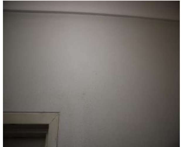
Figure 770 - Crack propagation through corridor internal wall
