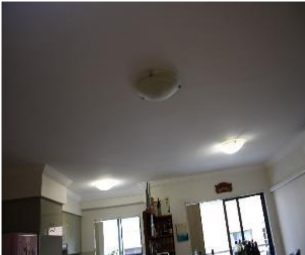
Figure 1117 - General condition of dining room ceiling
