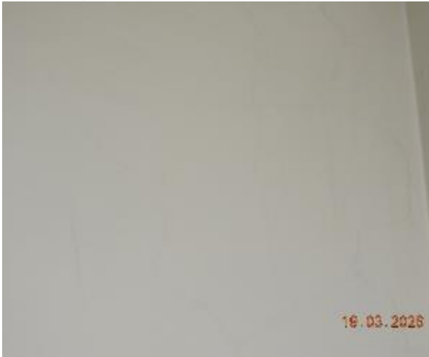
Figure 55 - Crack propagation through level 2 common area internal wall
