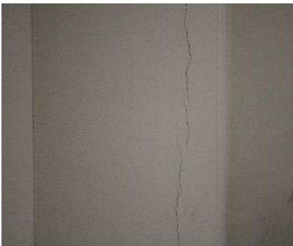
Figure 1272 - Crack propagation through lounge room internal wall
