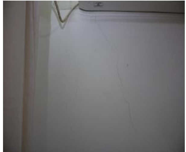
Figure 528 - Crack propagation through open kitchen/ lounge room internal wall
