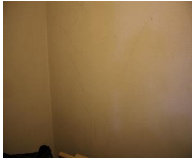
Figure 572 - Crack propagation through laundry internal wall
