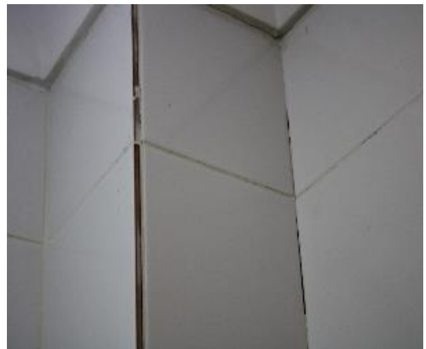
Figure 1403 - Crack propagation through ensuite bathroom internal wall
