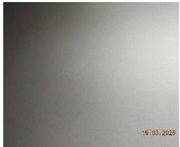
Figure 449 - Crack propagation through basement fire stairs internal wall
