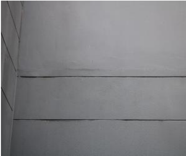
Figure 599 - Crack propagation through external wall
