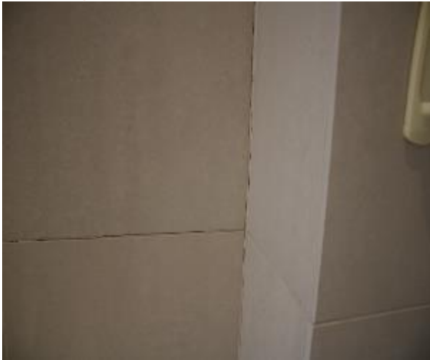
Figure 1014 - Crack propagation through bathroom 1 internal wall
