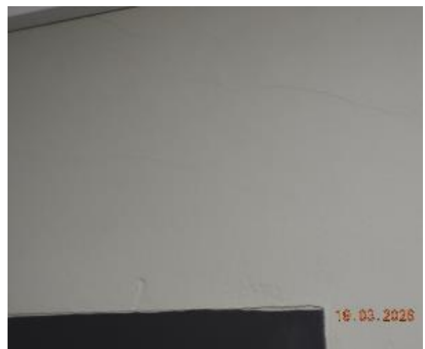
Figure 84 - Crack propagation through level 3 common area internal wall
