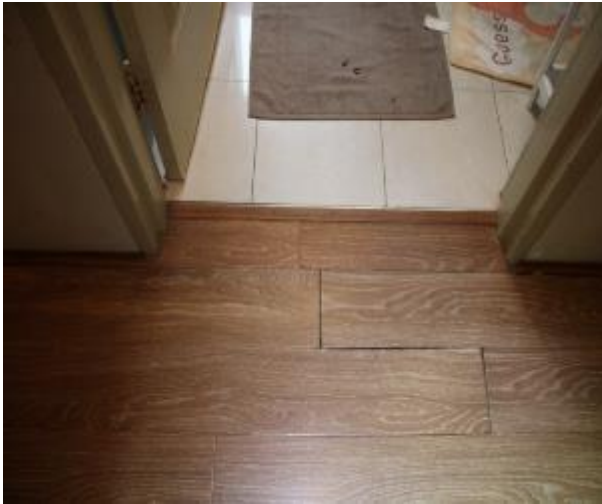
Figure 1340 - Displacement evident through corridor flooring
