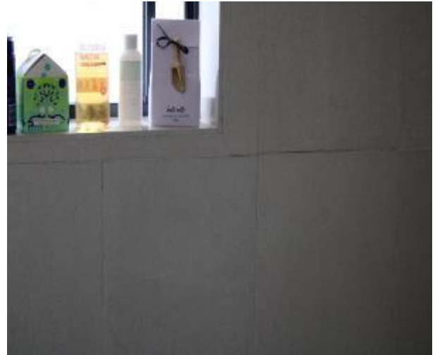
Figure 1164 - Crack propagation through bathroom 1 internal wall
