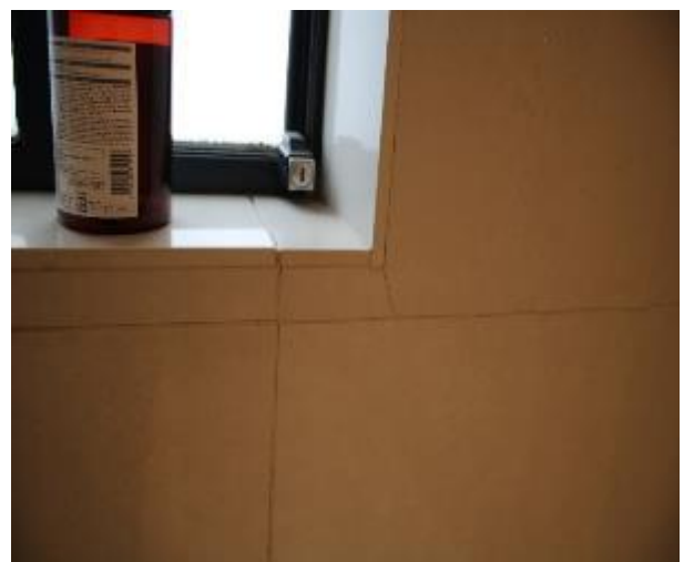
Figure 1001 - Crack propagation through bathroom 1 internal wall
