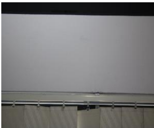
Figure 1549 - Crack propagation through bedroom 1 internal wall
