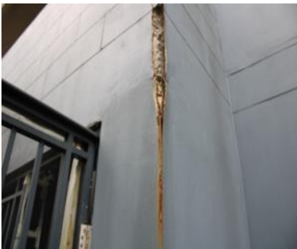
Figure 597 - Water damage evident through external wall
