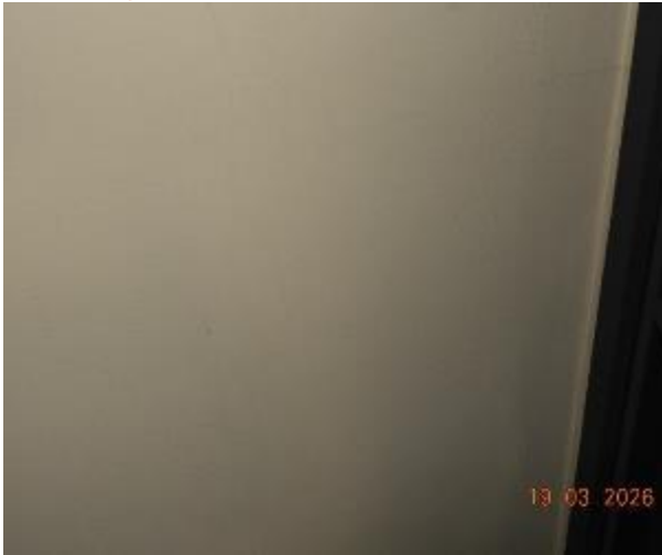
Figure 127 - Crack propagation through level 4 common area internal wall
