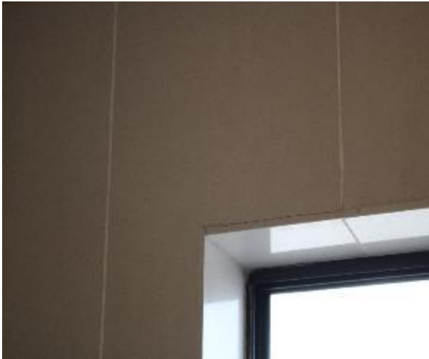
Figure 1364 - Crack propagation through bathroom 1 internal wall
