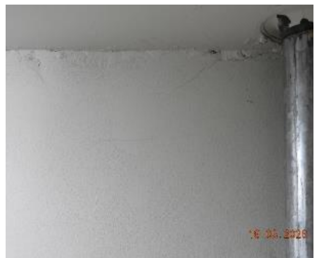
Figure 371 - Crack propagation through level 2 fire stairs internal wall
