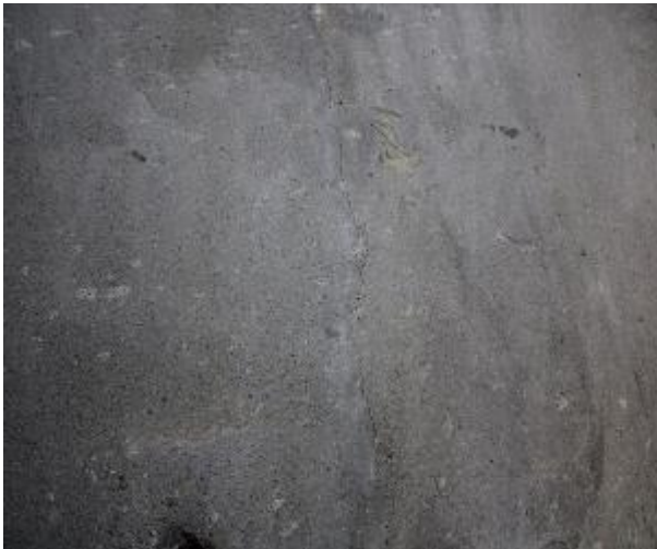
Figure 223 - Crack propagation through B1 fire stairs internal wall
