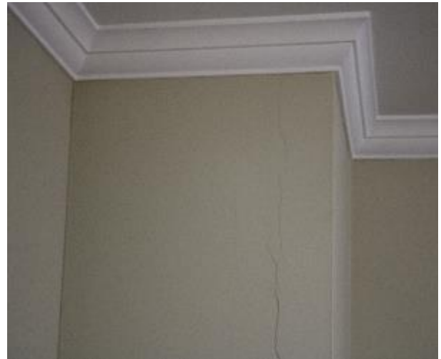
Figure 1271 - Crack propagation through lounge room internal wall
