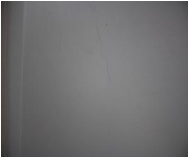
Figure 529 - Crack propagation through open kitchen/ lounge room internal wall
