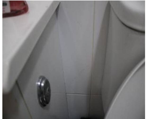
Figure 1212 - Crack propagation through ensuite bathroom internal wall
