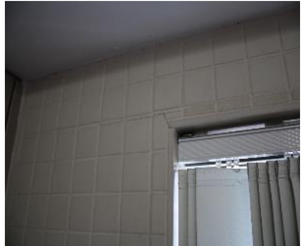
Figure 967 - Crack propagation through kitchen internal wall
