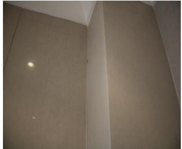
Figure 1015 - Crack propagation through bathroom 1 internal wall
