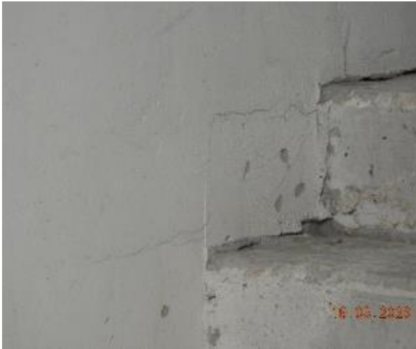
Figure 348 - Crack propagation through level 3 fire stairs internal wall
