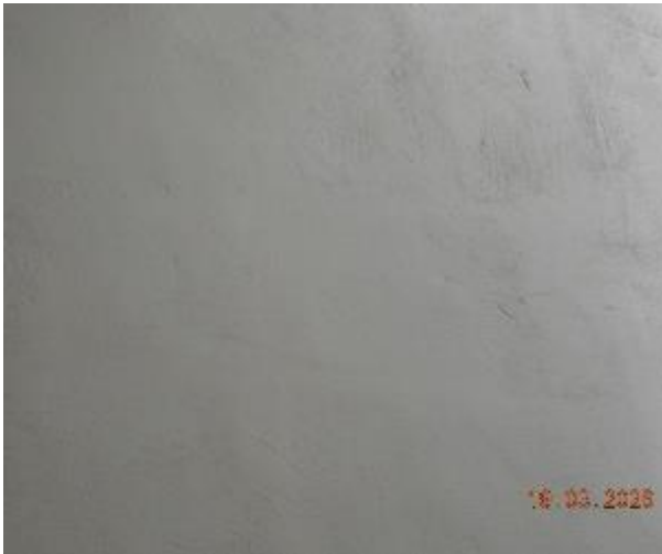
Figure 296 - Crack propagation through level 5 fire stairs internal wall
