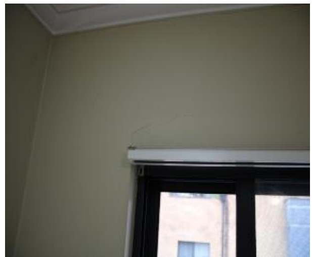
Figure 1285 - Crack propagation through lounge room internal wall
