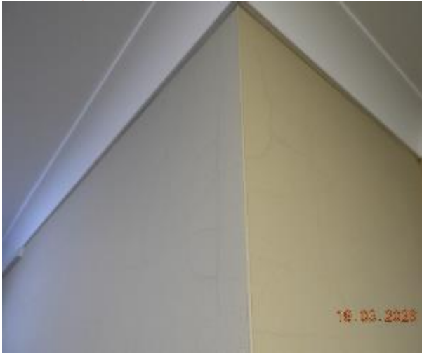
Figure 121 - Crack propagation through level 4 common area internal wall
