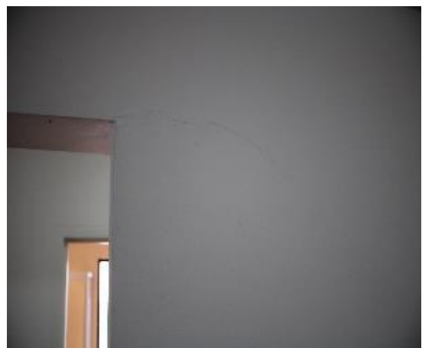
Figure 941 - Crack propagation through lounge room internal wall
