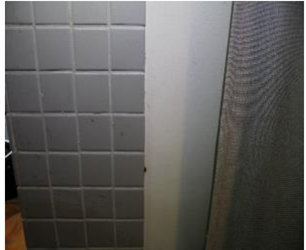
Figure 746 - Crack propagation through open kitchen/ lounge room internal wall
