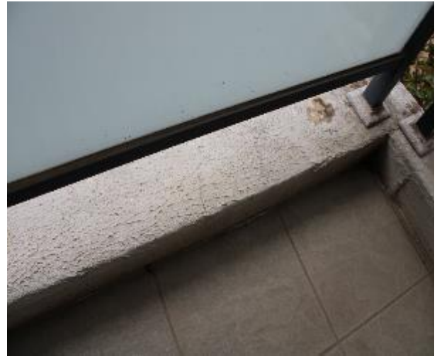
Figure 830 - Crack propagation through external wall
