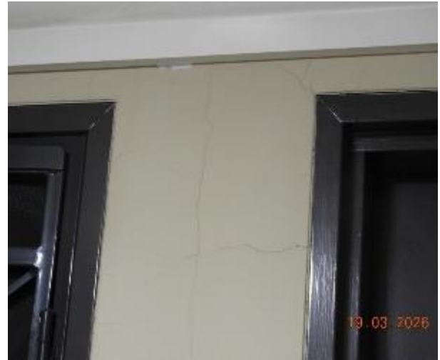
Figure 176 - Crack propagation through level 5 common area internal wall
