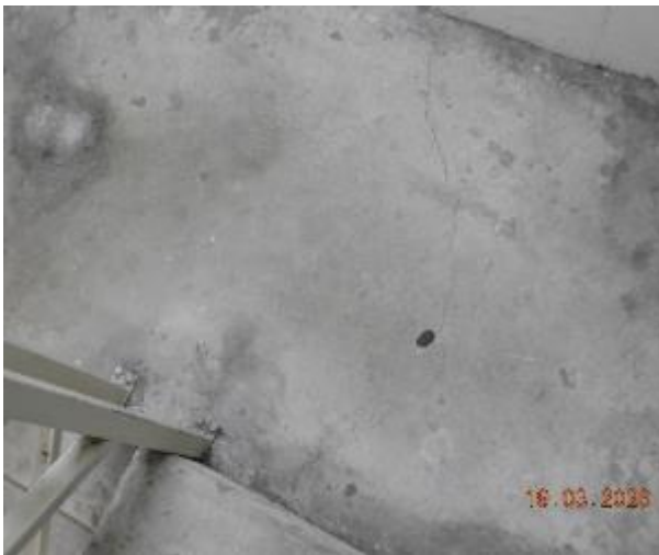
Figure 362 - Crack propagation through level 2 fire stairs concrete floor
