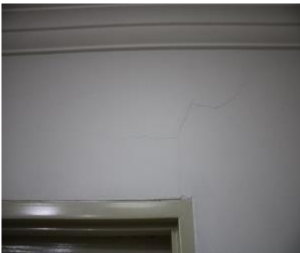
Figure 537 - Crack propagation through open kitchen/ lounge room internal wall
