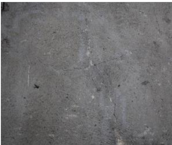
Figure 225 - Crack propagation through B1 fire stairs internal wall
