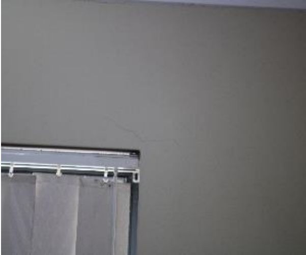
Figure 1418 - Crack propagation through study internal wall
