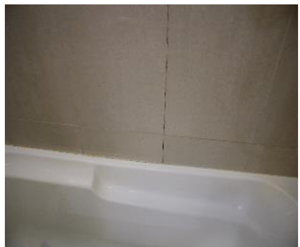
Figure 562 - Crack propagation through bathroom 1 internal wall
