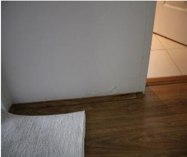
Figure 984 - Paint flaking through corridor internal wall
