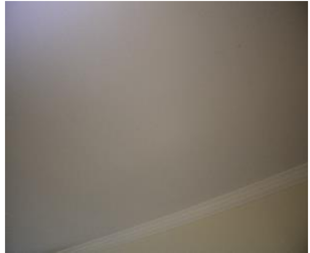
Figure 1116 - General condition of dining room ceiling
