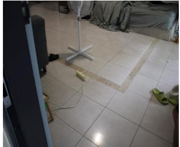
Figure 472 - General condition of open kitchen/ lounge room floor tiles
