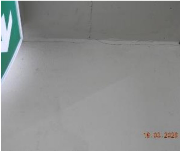
Figure 426 - Crack propagation through level 1 fire stairs internal wall
