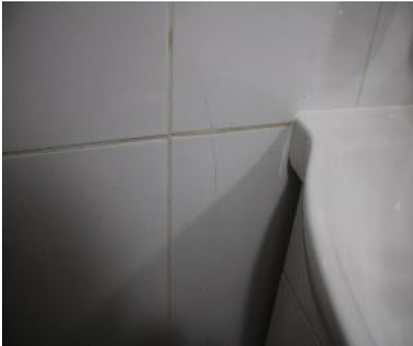
Figure 721 - Crack propagation through ensuite bathroom internal wall
