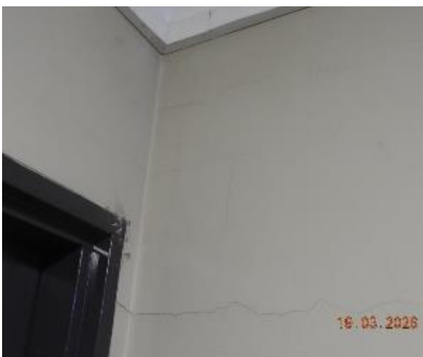
Figure 137 - Crack propagation through level 4 common area internal wall
