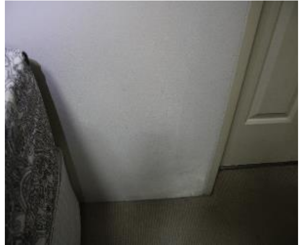
Figure 790 - Crack propagation through bedroom 1 internal wall
