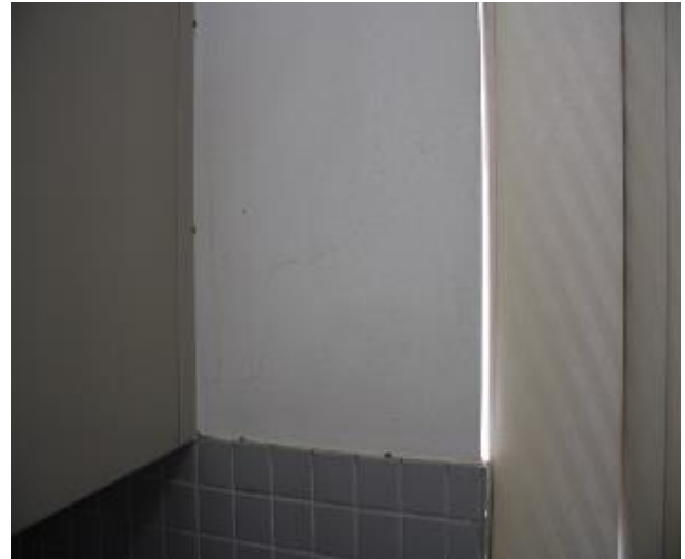
Figure 752 - Crack propagation through open kitchen/ lounge room internal wall
