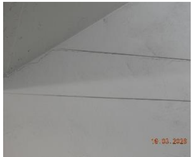
Figure 387 - Crack propagation through level 2 fire stairs internal wall
