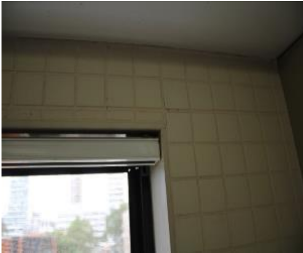
Figure 966 - Crack propagation through kitchen internal wall
