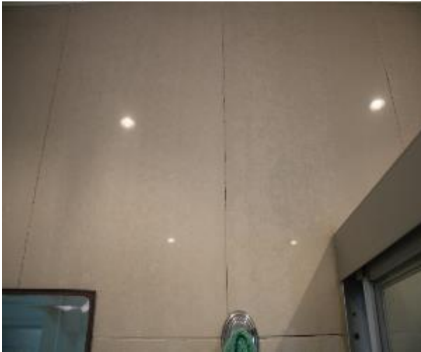
Figure 1020 - Crack propagation through bathroom 1 internal wall
