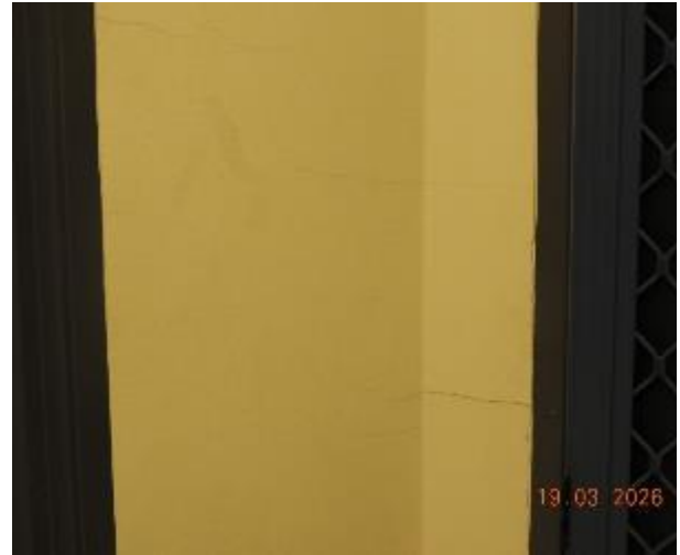
Figure 92 - Crack propagation through level 3 common area internal wall
