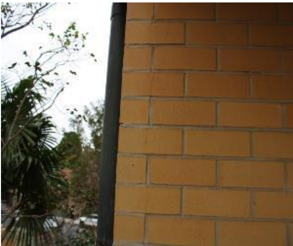
Figure 839 - Crack propagation through external wall
