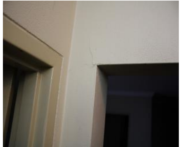
Figure 1335 - Crack propagation through corridor internal wall
