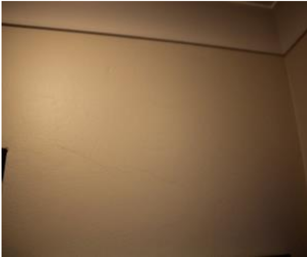
Figure 1151 - Crack propagation through corridor internal wall
