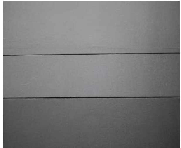
Figure 508 - Crack propagation through external wall
