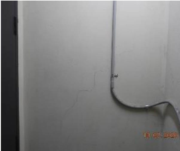
Figure 432 - Crack propagation through level 1 fire stairs internal wall
