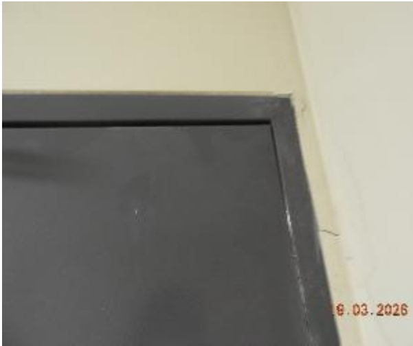
Figure 25 - Crack propagation through level 1 common area internal wall
