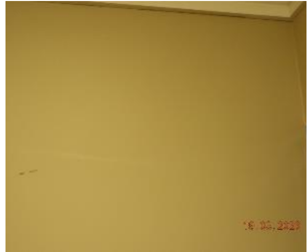
Figure 86 - Crack propagation through level 3 common area internal wall
