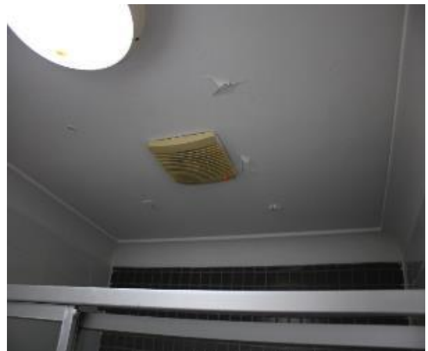
Figure 1226 - Paint flaking through ensuite bathroom ceiling
