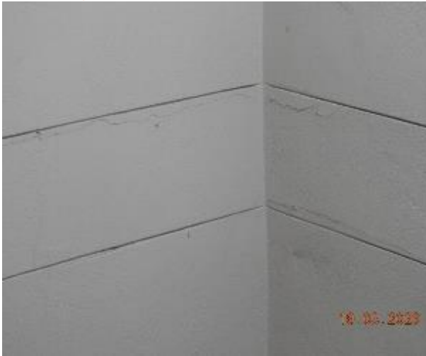
Figure 372 - Crack propagation through level 2 fire stairs internal wall
