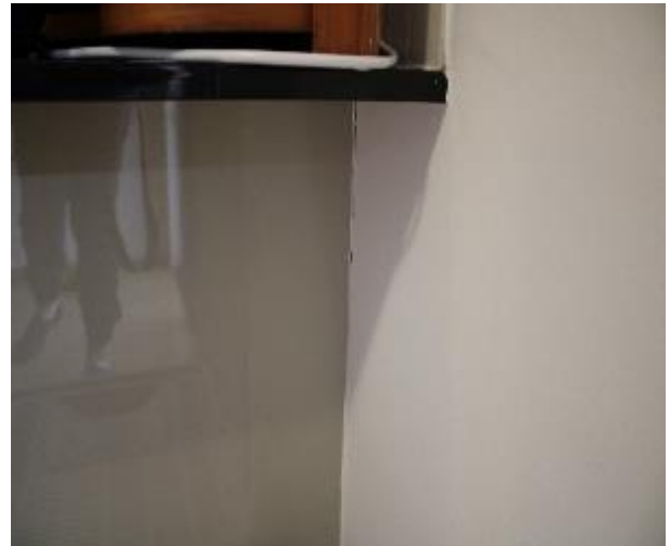
Figure 1112 - Crack propagation through dining room internal wall
