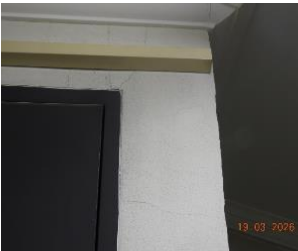
Figure 280 - Crack propagation through level 5 fire stairs internal wall
