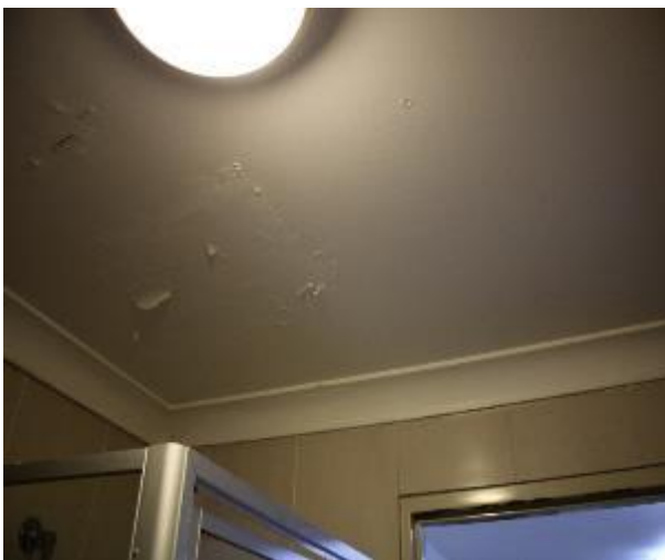
Figure 567 - Paint flaking through bathroom 1 ceiling
