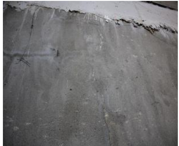
Figure 224 - Crack propagation through B1 fire stairs internal wall
