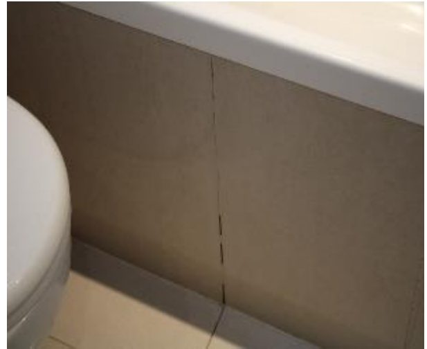
Figure 1009 - Crack propagation through bathroom 1 internal wall
