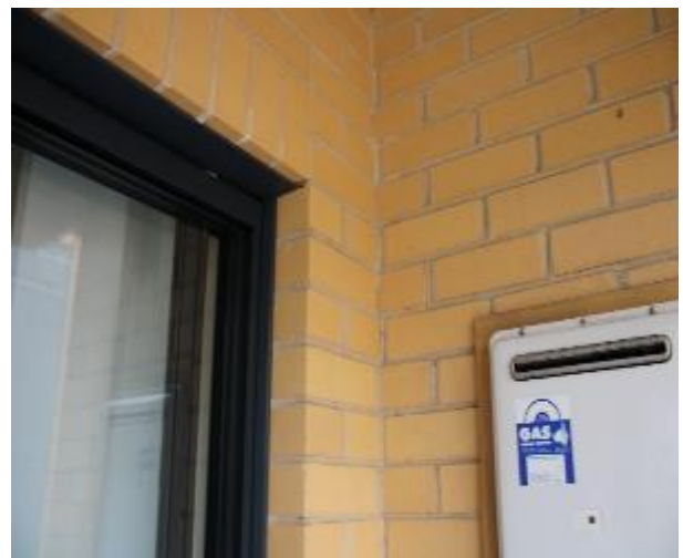
Figure 834 - Crack propagation through external wall
