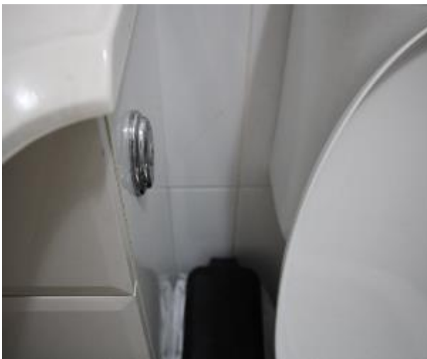
Figure 1213 - Crack propagation through ensuite bathroom internal wall
