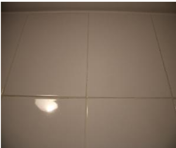
Figure 1627 - Crack propagation through ensuite bathroom internal wall
