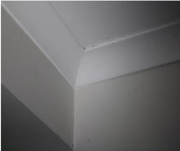
Figure 900 - Crack propagation through bedroom 2 ceiling
