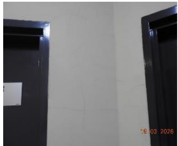
Figure 130 - Crack propagation through level 4 common area internal wall
