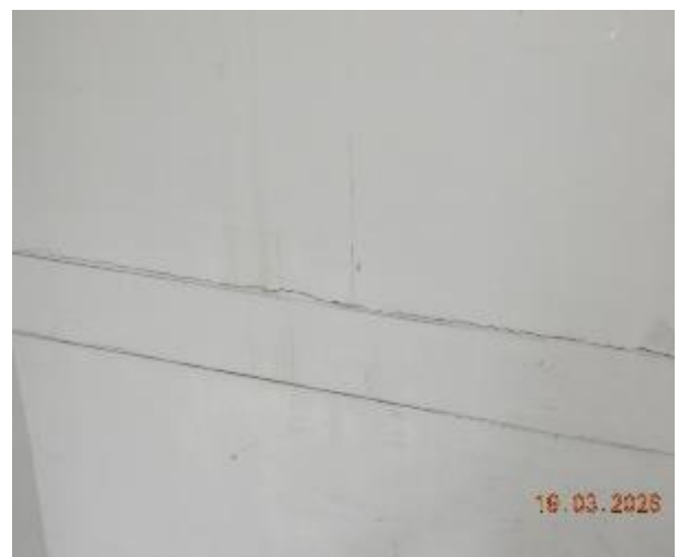
Figure 299 - Crack propagation through level 5 fire stairs internal wall
