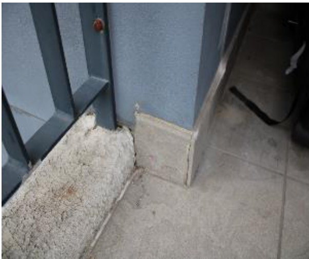
Figure 663 - Crack propagation through external wall
