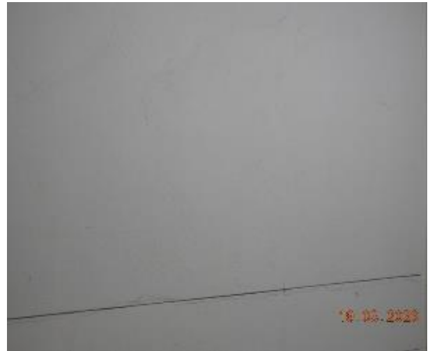
Figure 375 - Crack propagation through level 2 fire stairs internal wall
