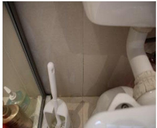
Figure 1007 - Crack propagation through bathroom 1 internal wall
