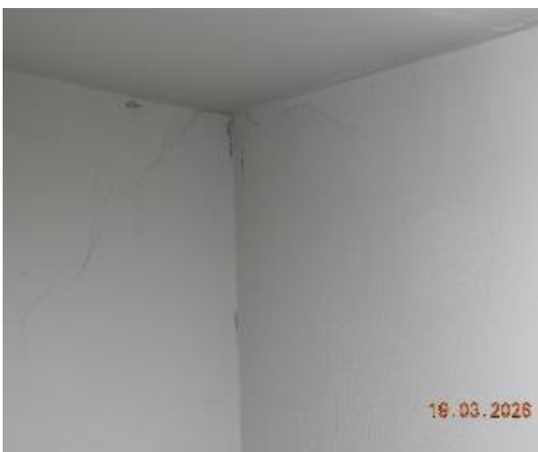
Figure 370 - Crack propagation through level 2 fire stairs internal wall
