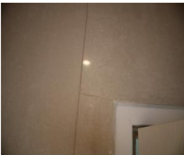
Figure 1018 - Crack propagation through bathroom 1 internal wall
