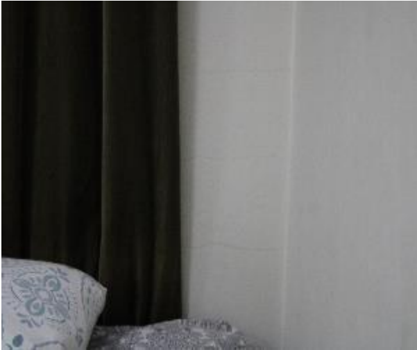
Figure 795 - Crack propagation through bedroom 1 internal wall
