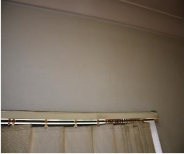
Figure 817 - Crack propagation through study internal wall
