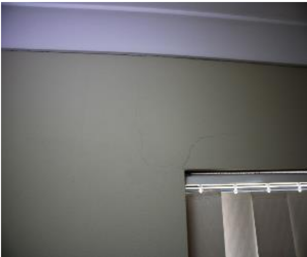
Figure 1420 - Crack propagation through study internal wall
