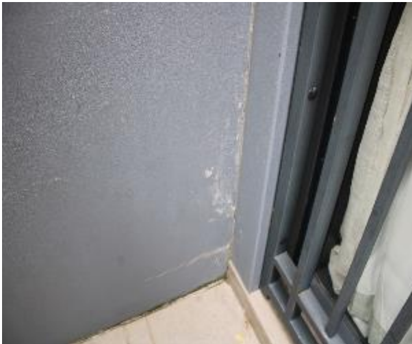
Figure 607 - Crack propagation through courtyard external wall
