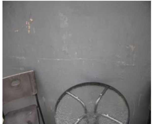
Figure 614 - Crack propagation through courtyard external wall
