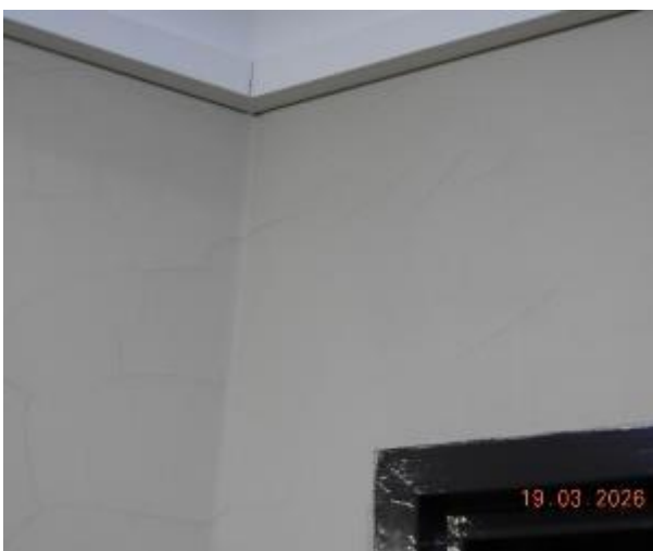
Figure 131 - Crack propagation through level 4 common area internal wall
