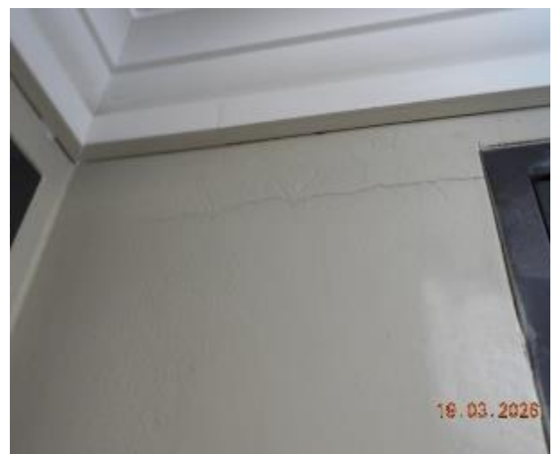
Figure 162 - Crack propagation through level 5 common area internal wall
