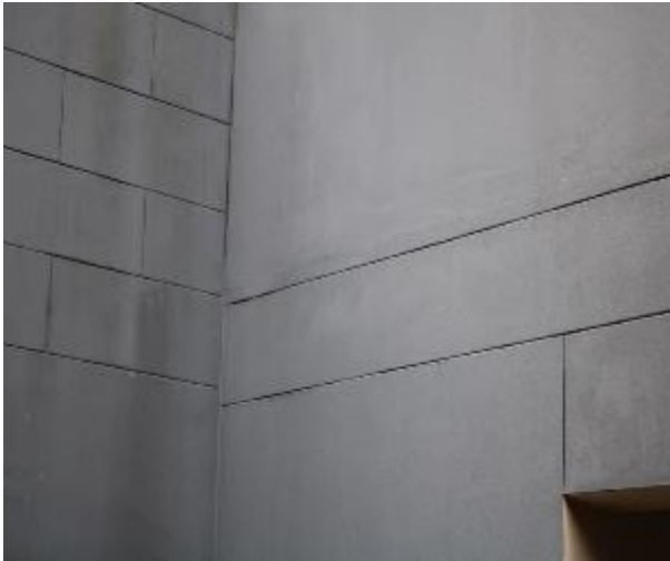
Figure 507 - Crack propagation through external wall
