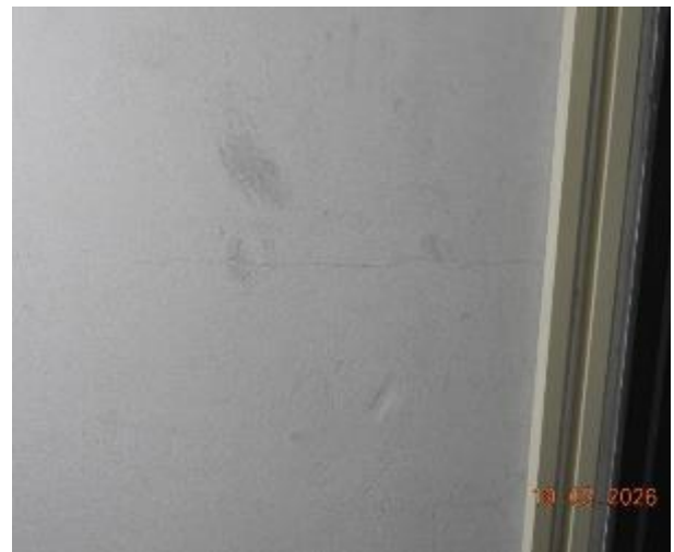
Figure 429 - Crack propagation through level 1 fire stairs internal wall
