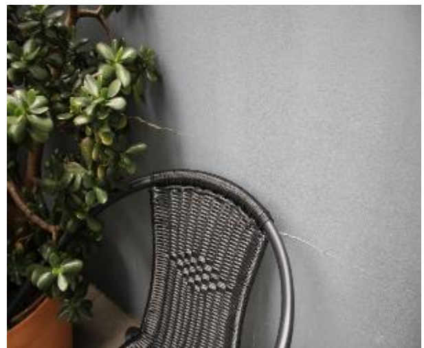
Figure 610 - Crack propagation through courtyard external wall
