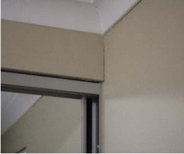
Figure 1370 - Crack propagation through bedroom 1 internal wall
