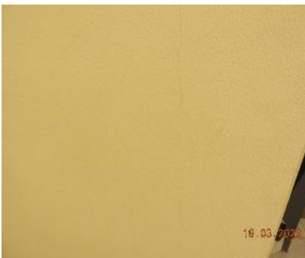
Figure 83 - Crack propagation through level 3 common area internal wall
