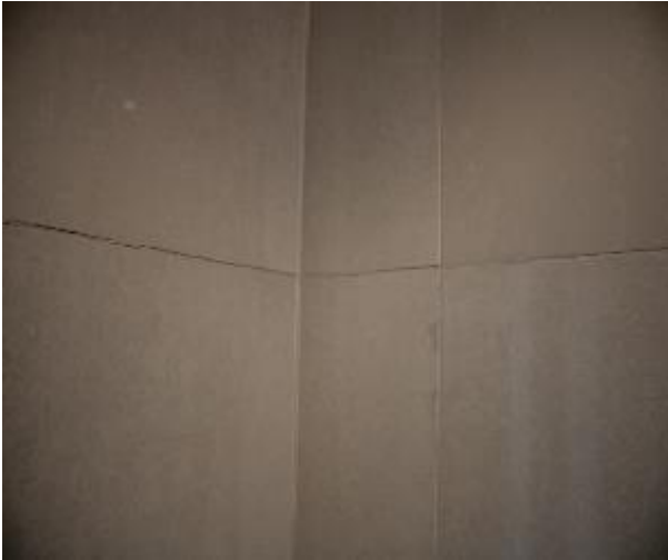
Figure 1004 - Crack propagation through bathroom 1 internal wall
