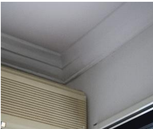
Figure 1479 - Crack propagation through open kitchen/ lounge room ceiling
