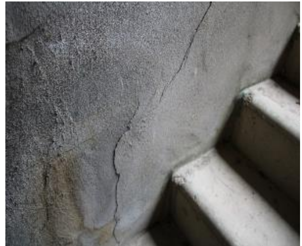
Figure 260 - Crack propagation through level 1 fire stairs internal wall
