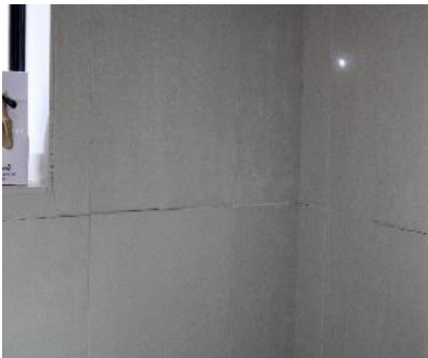
Figure 1165 - Crack propagation through bathroom 1 internal wall
