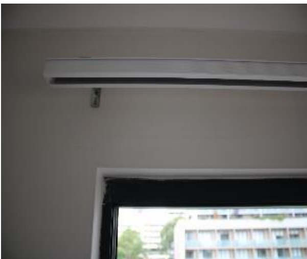
Figure 1060 - Crack propagation through bedroom 2 internal wall
