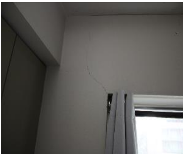
Figure 647 - Crack propagation through kitchen internal wall
