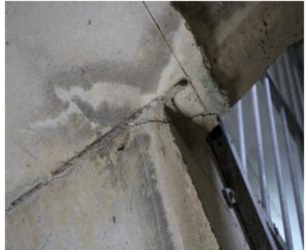
Figure 210 - Crack propagation through B2 fire stairs underside stairs
