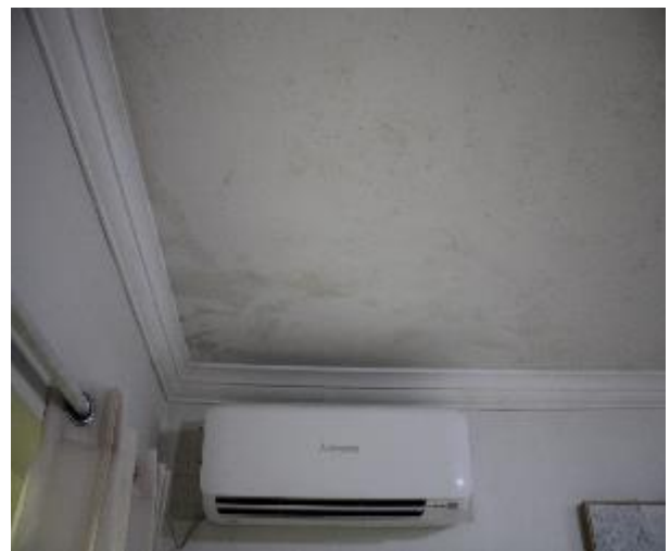
Figure 544 - Water damage evident through open kitchen/ lounge room ceiling
