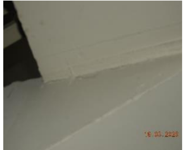
Figure 343 - Crack propagation through level 3 fire stairs underside stairs
