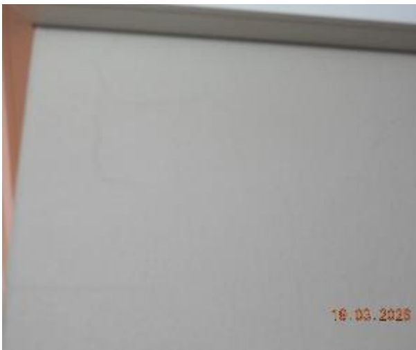
Figure 165 - Crack propagation through level 5 common area internal wall
