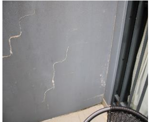
Figure 606 - Crack propagation through courtyard external wall
