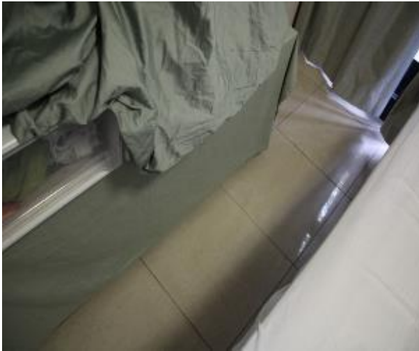
Figure 551 - General condition of bedroom 1 floor tiles
