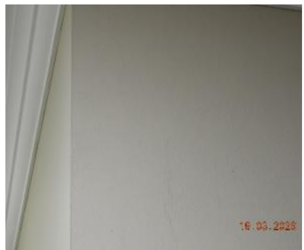
Figure 108 - Crack propagation through level 3 common area internal wall
