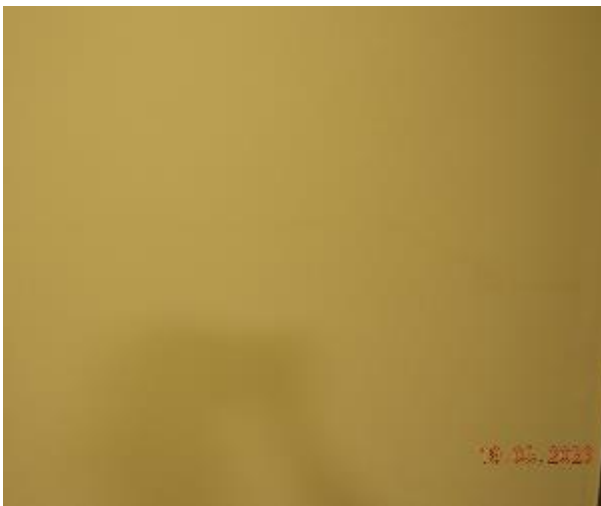
Figure 87 - Crack propagation through level 3 common area internal wall
