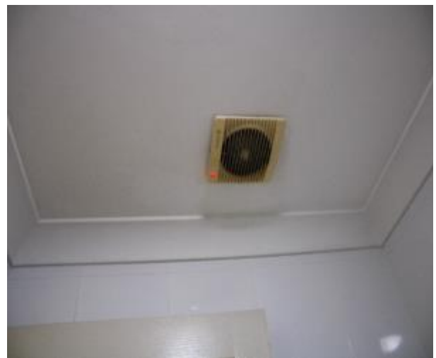
Figure 726 - General condition of ensuite bathroom ceiling
