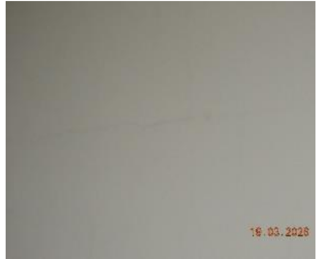
Figure 170 - Crack propagation through level 5 common area internal wall
