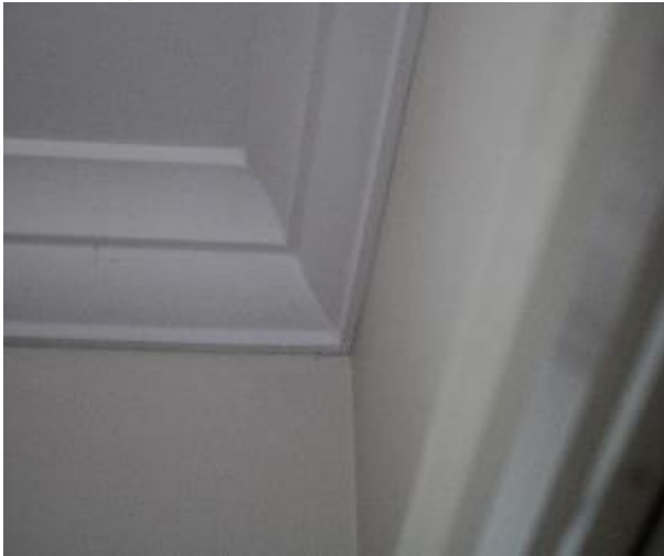
Figure 1121 - Crack propagation through dining room ceiling
