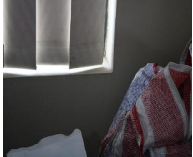
Figure 1419 - Crack propagation through study internal wall
