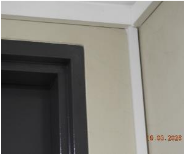
Figure 175 - Crack propagation through level 5 common area internal wall
