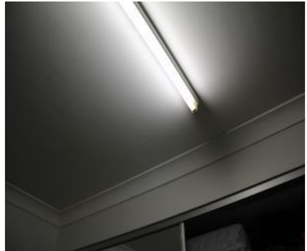
Figure 712 - General condition of dressing room ceiling
