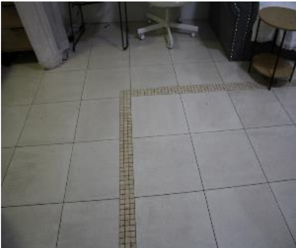
Figure 523 - General condition of open kitchen/ lounge room floor tiles
