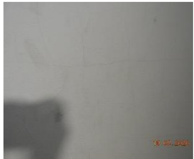
Figure 160 - Crack propagation through level 5 common area internal wall
