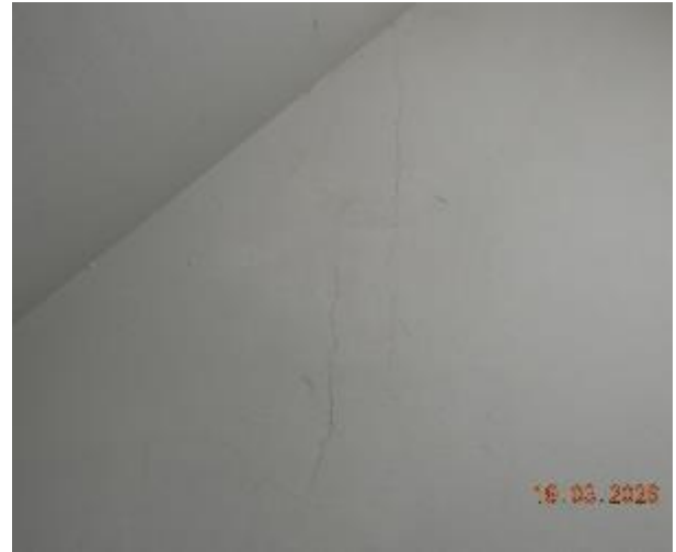
Figure 355 - Crack propagation through level 3 fire stairs internal wall
