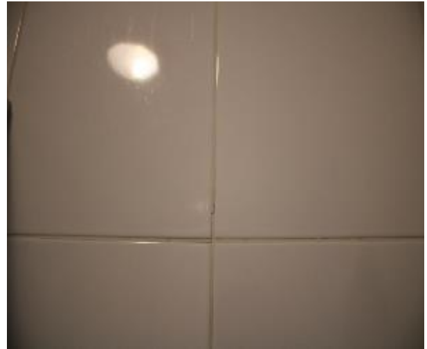
Figure 1626 - Crack propagation through ensuite bathroom internal wall
