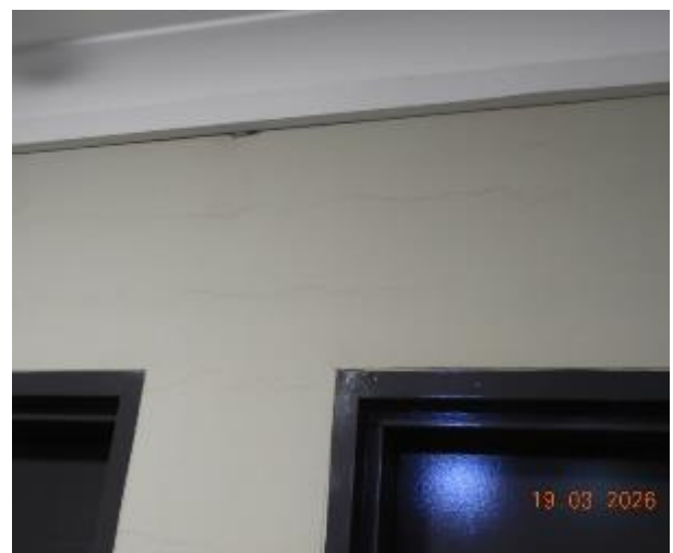
Figure 138 - Crack propagation through level 4 common area internal wall
