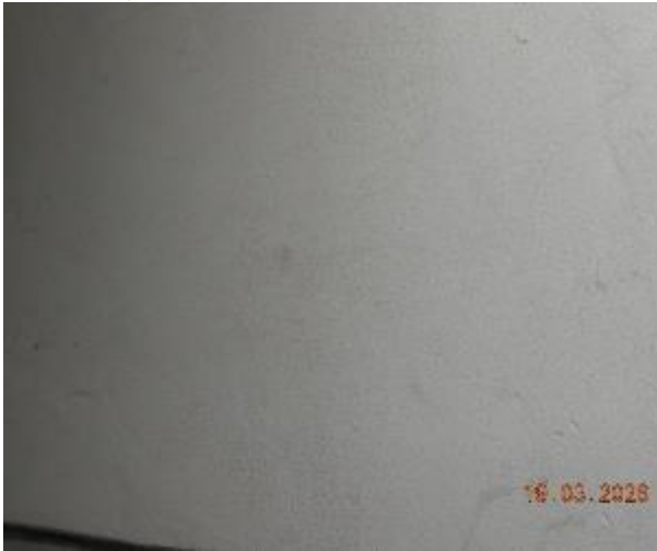
Figure 450 - Crack propagation through basement fire stairs internal wall
