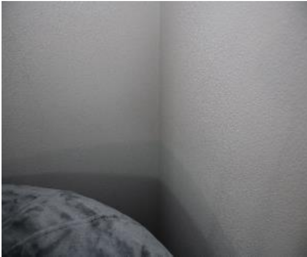
Figure 631 - Crack propagation through lounge room internal wall
