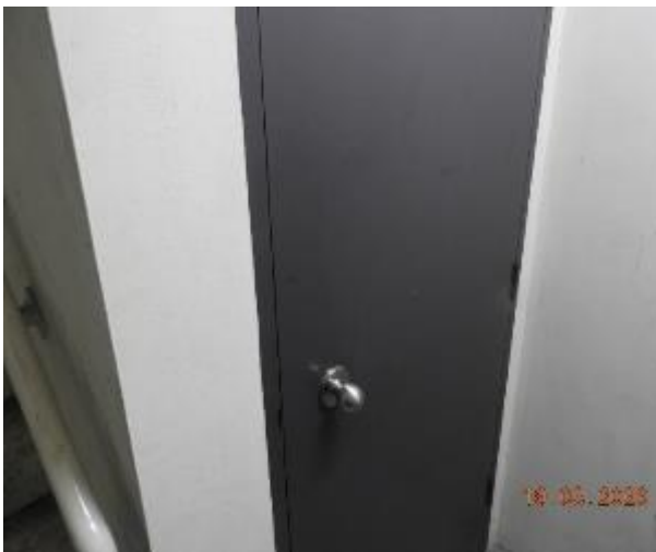
Figure 440 - The following images display the condition of the basement fire stairs
