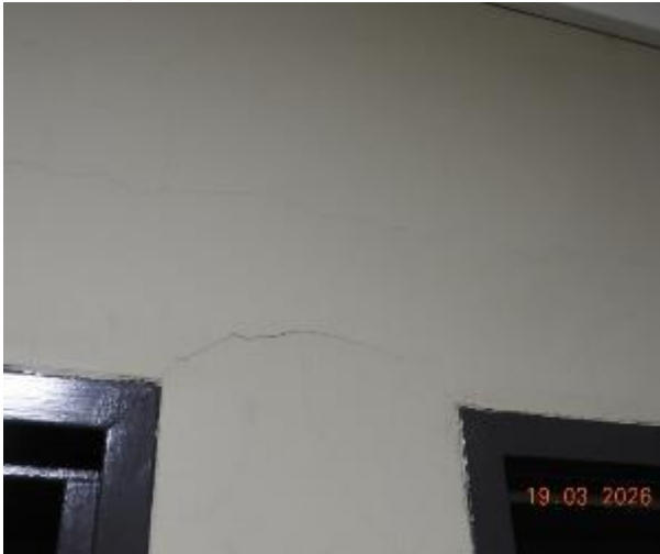
Figure 67 - Crack propagation through level 2 common area internal wall
