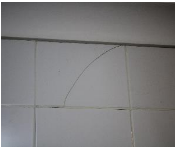
Figure 1402 - Crack propagation through ensuite bathroom internal wall
