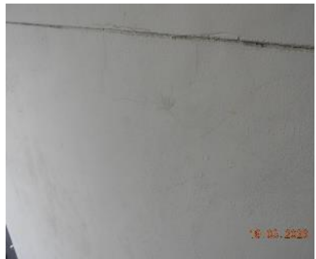
Figure 305 - Crack propagation through level 5 fire stairs internal wall
