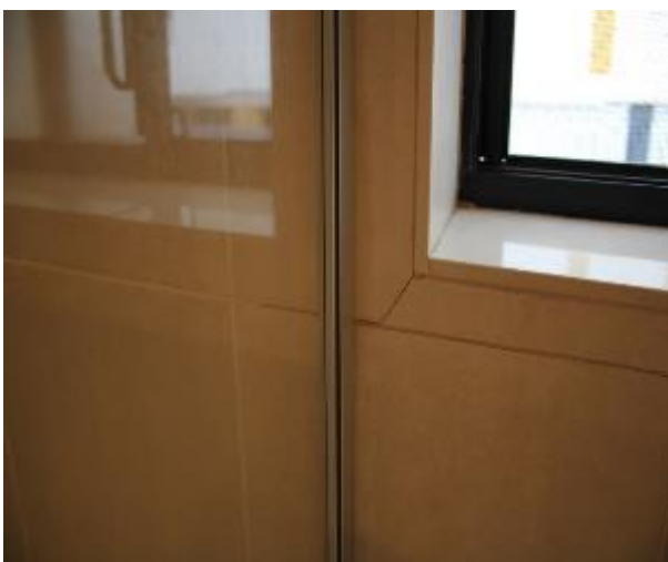
Figure 1000 - Crack propagation through bathroom 1 internal wall
