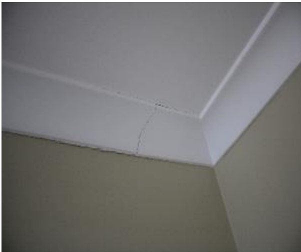
Figure 1426 - Crack propagation through study ceiling
