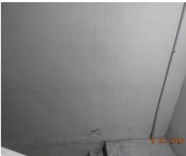
Figure 322 - Crack propagation through level 4 fire stairs internal wall
