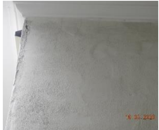
Figure 309 - Crack propagation through level 5 fire stairs internal wall
