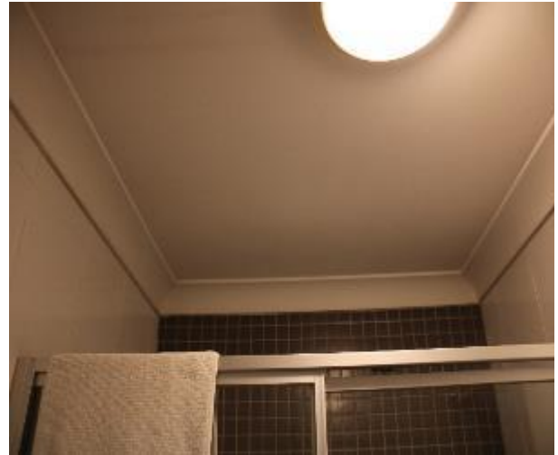
Figure 812 - General condition of ensuite bathroom ceiling
