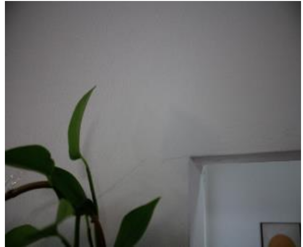
Figure 955 - Crack propagation through lounge room internal wall
