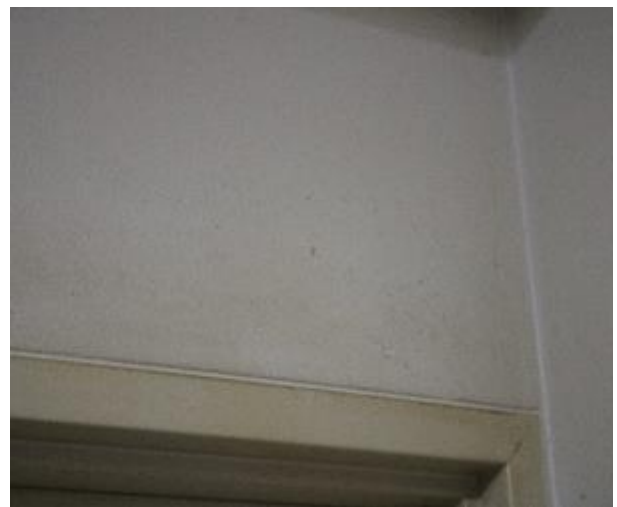
Figure 792 - Crack propagation through bedroom 1 internal wall
