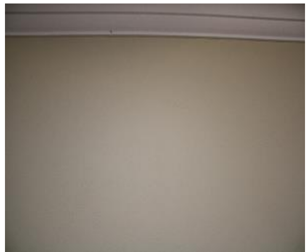
Figure 1291 - Crack propagation through lounge room internal wall
