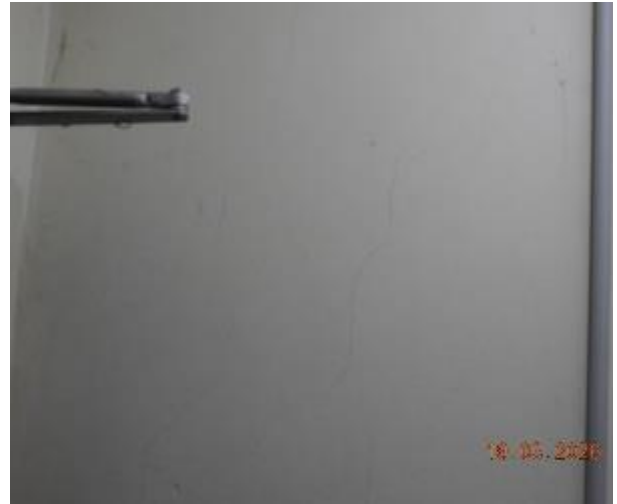
Figure 433 - Crack propagation through level 1 fire stairs internal wall
