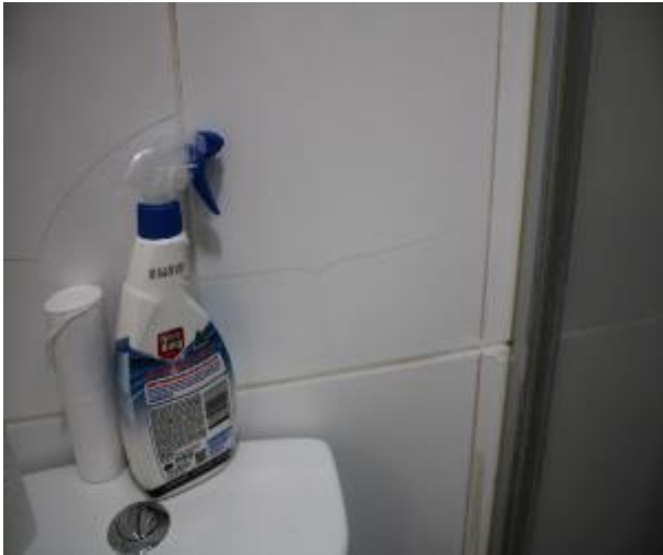
Figure 1211 - Crack propagation through ensuite bathroom internal wall
