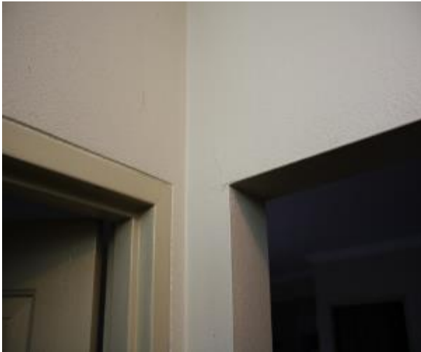
Figure 1334 - Crack propagation through corridor internal wall
