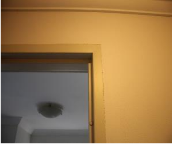
Figure 1493 - Crack propagation through laundry internal wall
