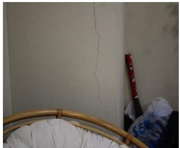
Figure 1273 - Crack propagation through lounge room internal wall
