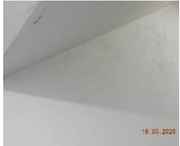
Figure 367 - Crack propagation through level 2 fire stairs internal wall
