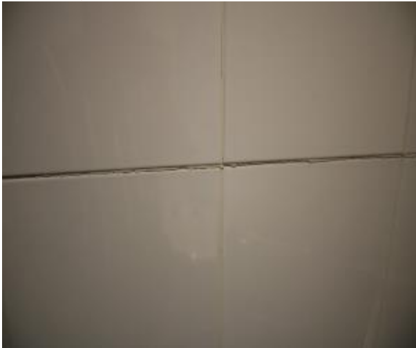
Figure 1050 - Crack propagation through ensuite bathroom internal wall
