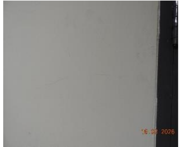
Figure 26 - Crack propagation through level 1 common area internal wall
