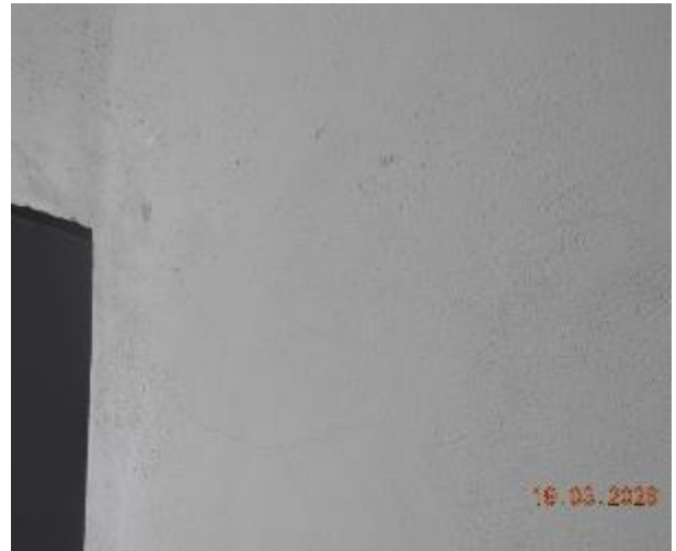
Figure 315 - Crack propagation through level 4 fire stairs internal wall
