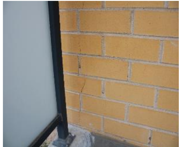
Figure 838 - Crack propagation through external wall
