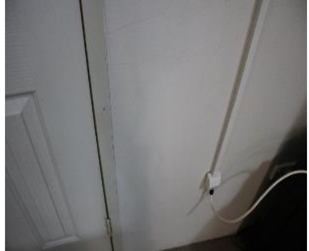
Figure 734 - Crack propagation through open kitchen/ lounge room internal wall
