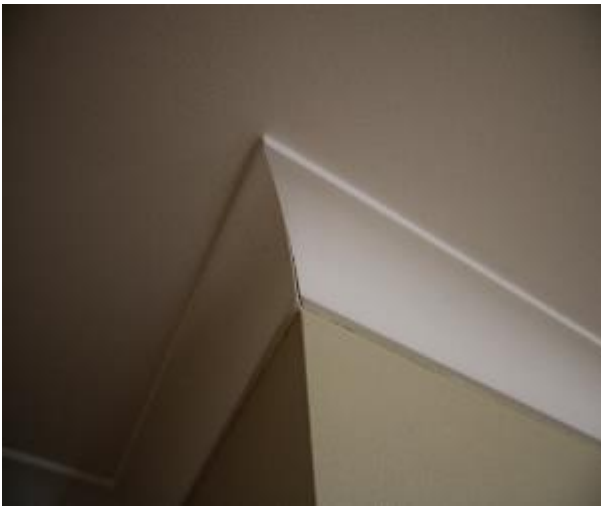
Figure 1384 - Crack propagation through bedroom 1 ceiling
