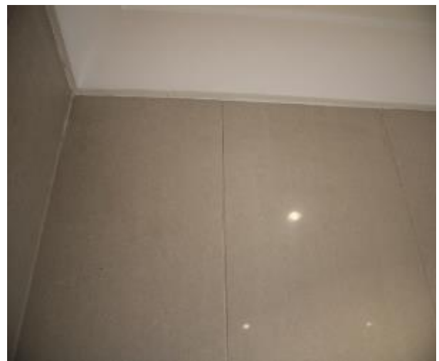
Figure 995 - Crack propagation through bathroom 1 internal wall
