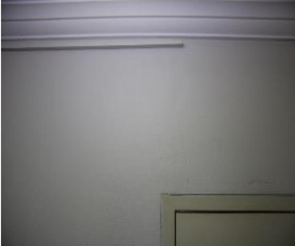
Figure 733 - Crack propagation through open kitchen/ lounge room internal wall
