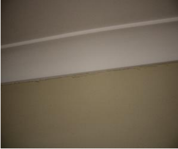
Figure 1388 - Crack propagation through bedroom 1 ceiling
