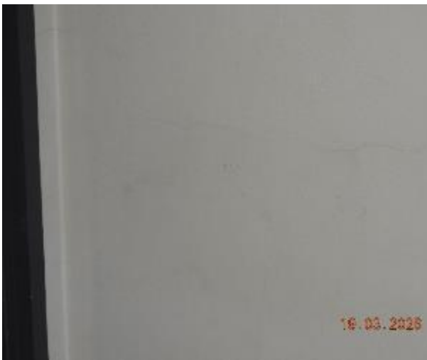
Figure 135 - Crack propagation through level 4 common area internal wall
