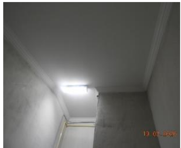
Figure 311 - General condition of level 5 fire stairs ceiling
