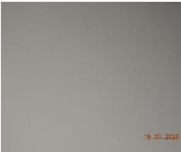
Figure 171 - Crack propagation through level 5 common area internal wall
