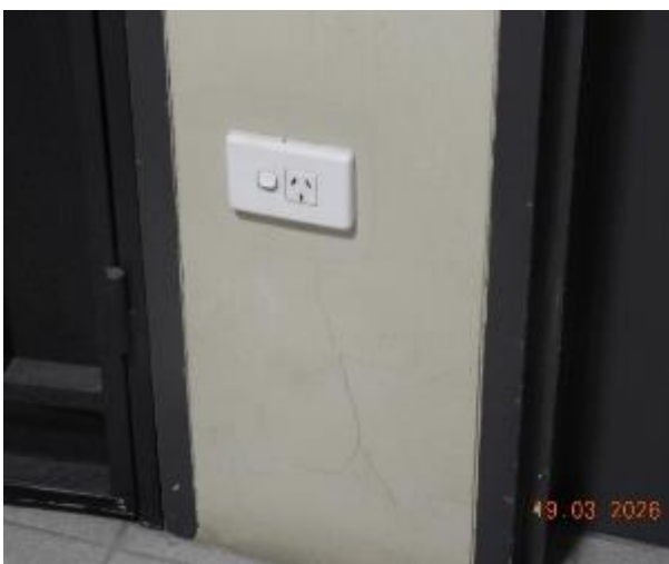
Figure 173 - Crack propagation through level 5 common area internal wall
