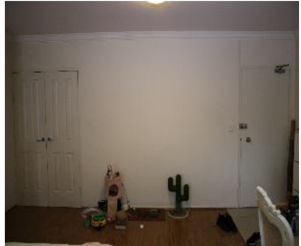
Figure 1098 - General condition of dining room internal wall
