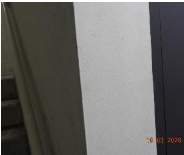
Figure 436 - Crack propagation through level 1 fire stairs internal wall
