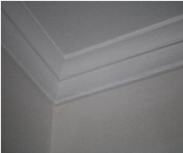
Figure 1477 - Crack propagation through open kitchen/ lounge room ceiling
