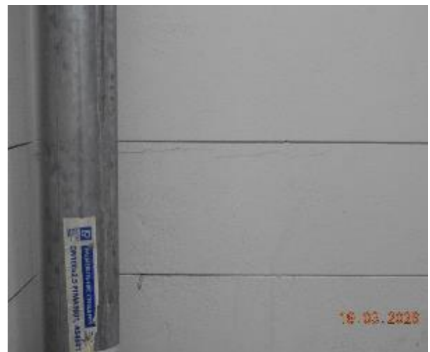
Figure 365 - Crack propagation through level 2 fire stairs internal wall
