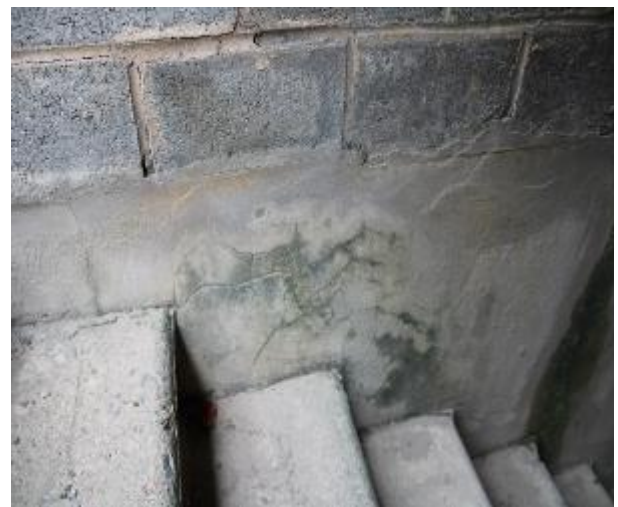
Figure 262 - Crack propagation through level 1 fire stairs internal wall
