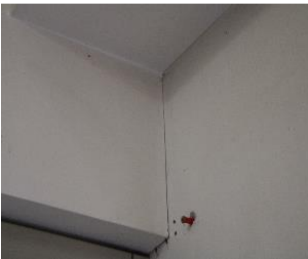
Figure 755 - Crack propagation through open kitchen/ lounge room internal wall
