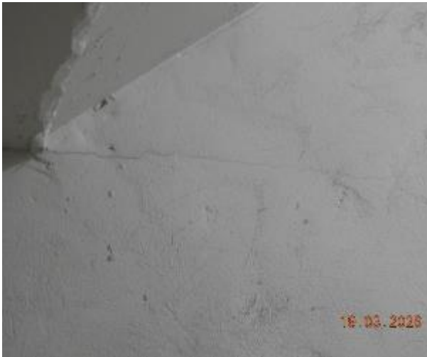
Figure 332 - Crack propagation through level 3 fire stairs internal wall
