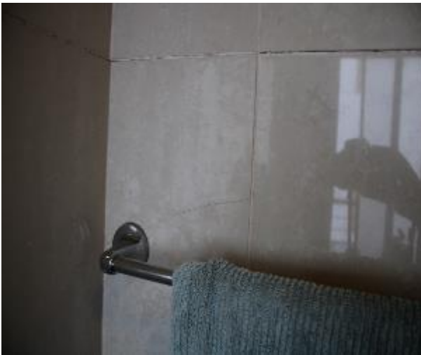
Figure 1597 - Crack propagation through bathroom 1 internal wall
