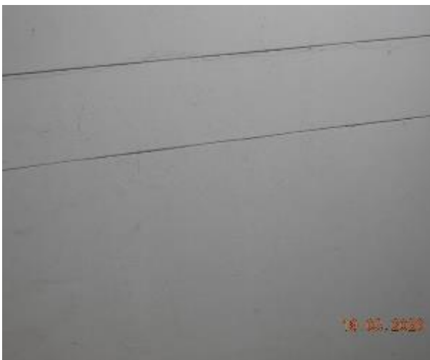
Figure 376 - Crack propagation through level 2 fire stairs internal wall
