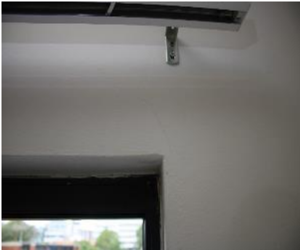
Figure 944 - Crack propagation through lounge room internal wall
