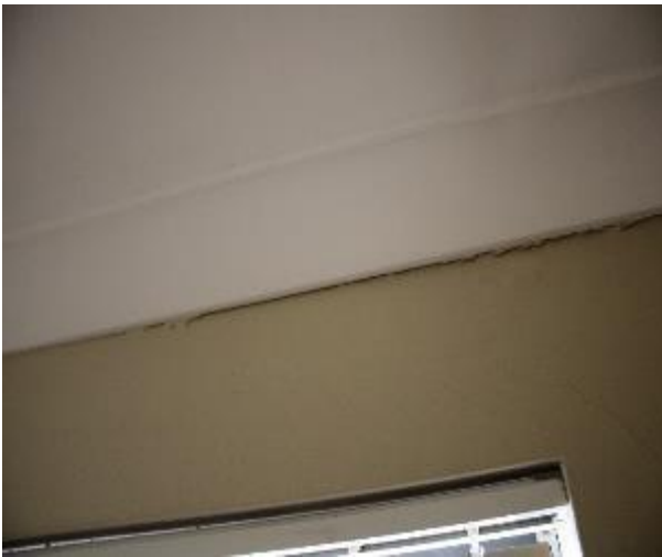
Figure 1390 - Crack propagation through bedroom 1 ceiling
