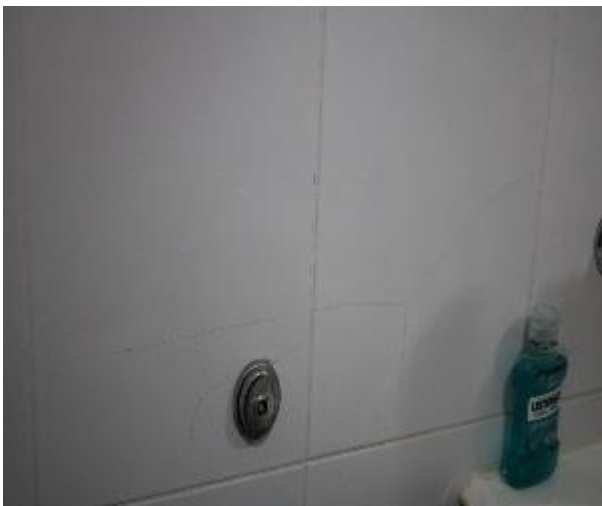
Figure 1219 - Crack propagation through ensuite bathroom internal wall
