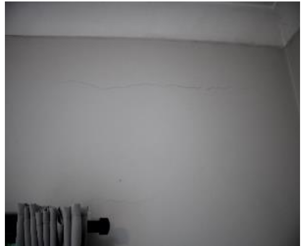
Figure 682 - Crack propagation through bedroom 1 internal wall
