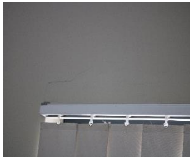
Figure 1415 - Crack propagation through study internal wall
