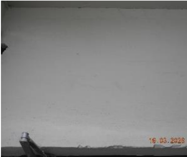
Figure 318 - Crack propagation through level 4 fire stairs internal wall
