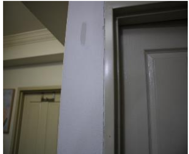
Figure 536 - Crack propagation through open kitchen/ lounge room internal wall
