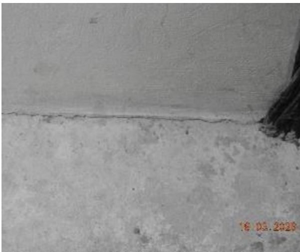
Figure 422 - Crack propagation through level 1 fire stairs concrete floor
