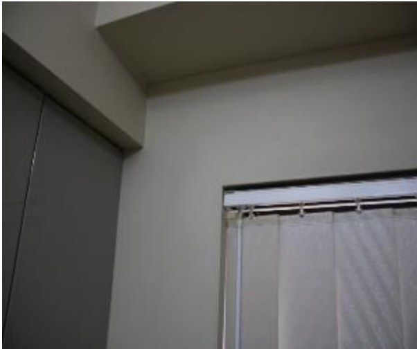
Figure 1310 - Crack propagation through kitchen internal wall
