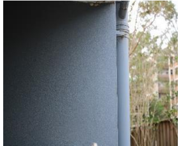
Figure 502 - Crack propagation through external wall
