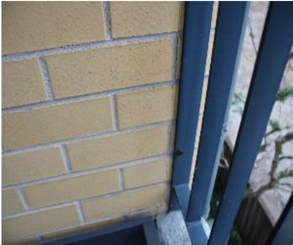
Figure 655 - Crack propagation through external wall
