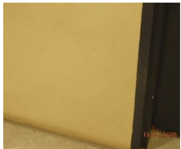
Figure 96 - Crack propagation through level 3 common area internal wall
