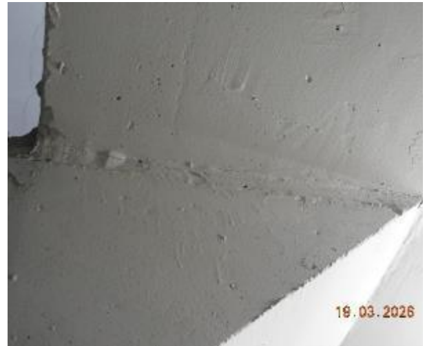
Figure 357 - Crack propagation through level 3 fire stairs underside stairs
