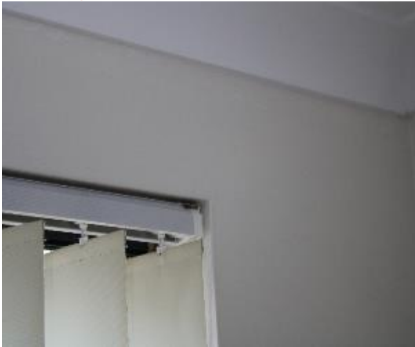
Figure 1187 - Crack propagation through bedroom 1 internal wall
