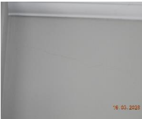
Figure 11 - Crack propagation through level 1 common area internal wall
