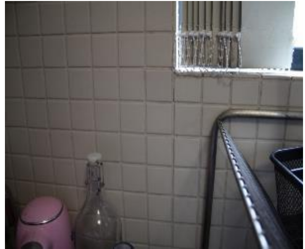
Figure 1128 - Crack propagation through kitchen internal wall
