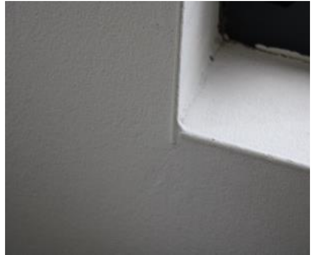
Figure 1188 - Crack propagation through bedroom 1 internal wall
