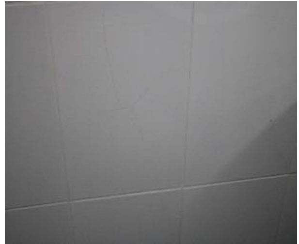
Figure 1218 - Crack propagation through ensuite bathroom internal wall
