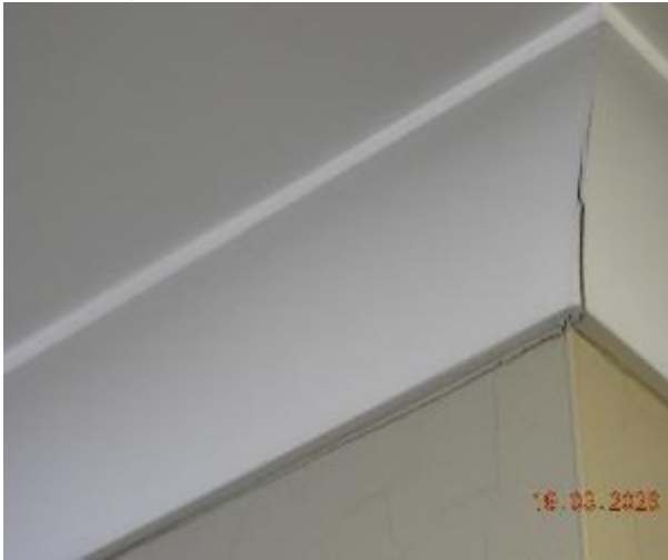
Figure 145 - Crack propagation through level 4 common area ceiling
