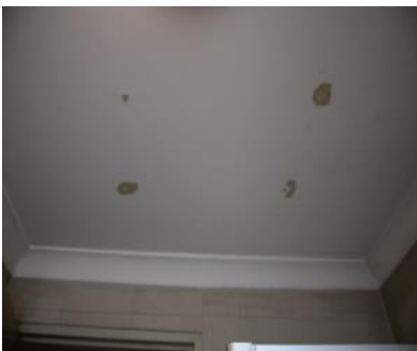
Figure 1542 - General condition of bathroom 1 ceiling
