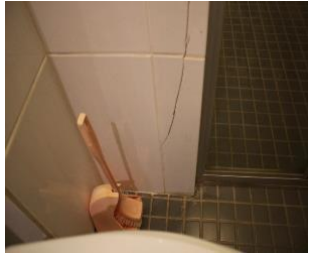
Figure 1147 - Crack propagation through ensuite bathroom internal wall
