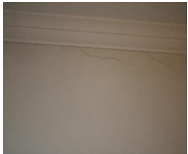
Figure 1103 - Crack propagation through lounge room internal wall
