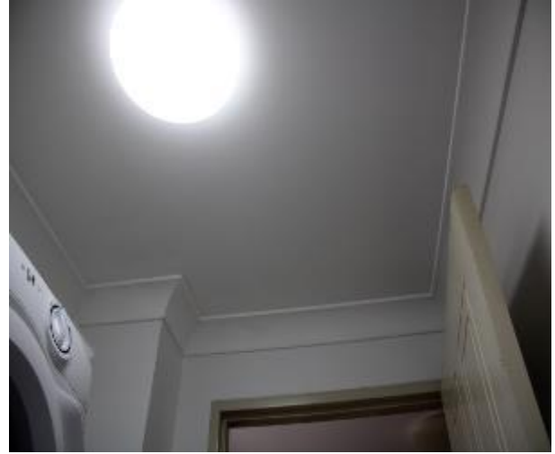
Figure 1267 - General condition of laundry ceiling
