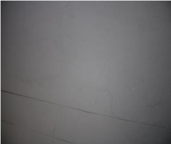
Figure 261 - Crack propagation through level 5 to basement B2 fire stairs internal wall
