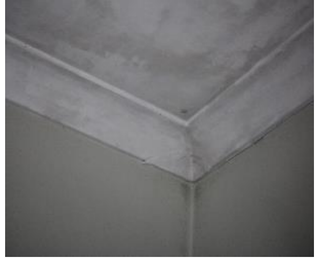
Figure 925 - Crack propagation through bedroom 3 ceiling
