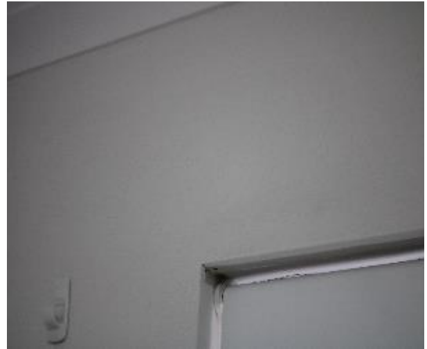
Figure 759 - Crack propagation through bedroom 3 internal wall
