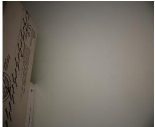
Figure 1203 - Crack propagation through study internal wall
