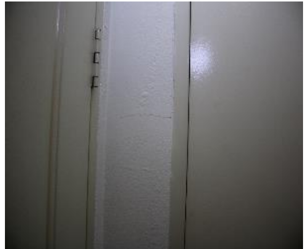
Figure 807 - Crack propagation through open kitchen/ lounge room internal wall
