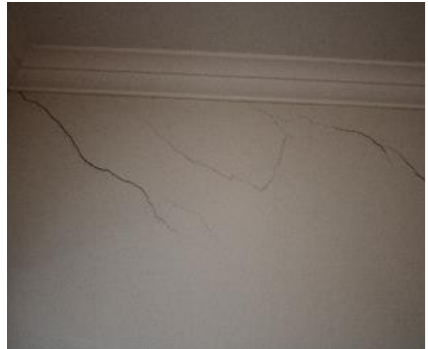
Figure 1101 - Crack propagation through lounge room internal wall
