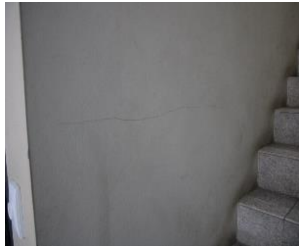
Figure 118 - Crack propagation through staircase to level 5 common area internal wall
