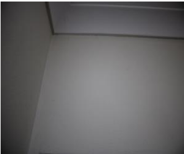
Figure 584 - Crack propagation through corridor internal wall
