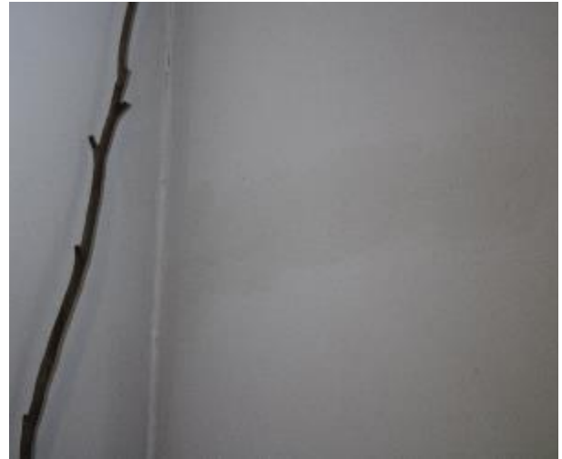
Figure 1551 - Crack propagation through bedroom 2 internal wall
