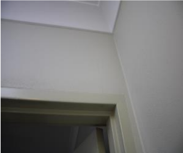
Figure 1468 - Crack propagation through corridor internal wall
