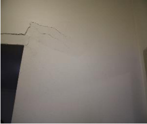
Figure 580 - Crack propagation through corridor internal wall
