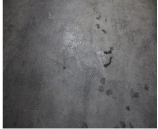
Figure 436 - Crack propagation through basement B2 fire stairs pavement slab
