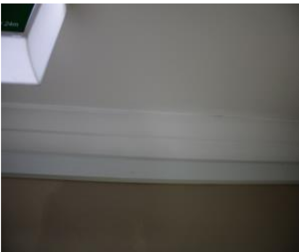
Figure 113 - Crack propagation through level 4 common area ceiling
