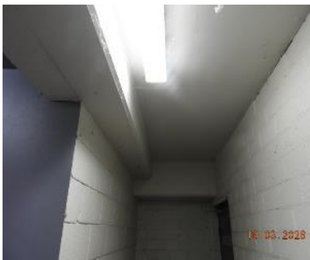
Figure 189 - General condition of B2 to Level 1 fire stairs underside slab
