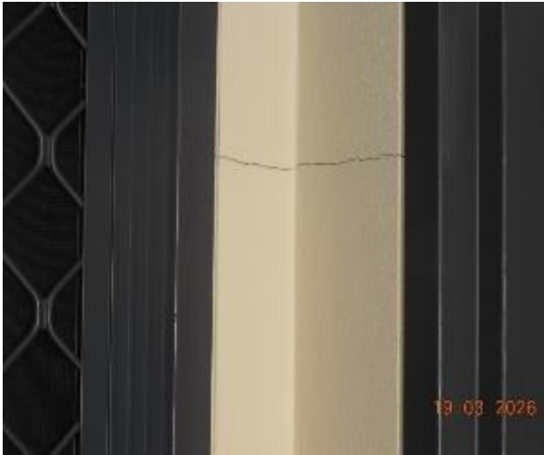
Figure 73 - Crack propagation through level 3 common area internal wall
