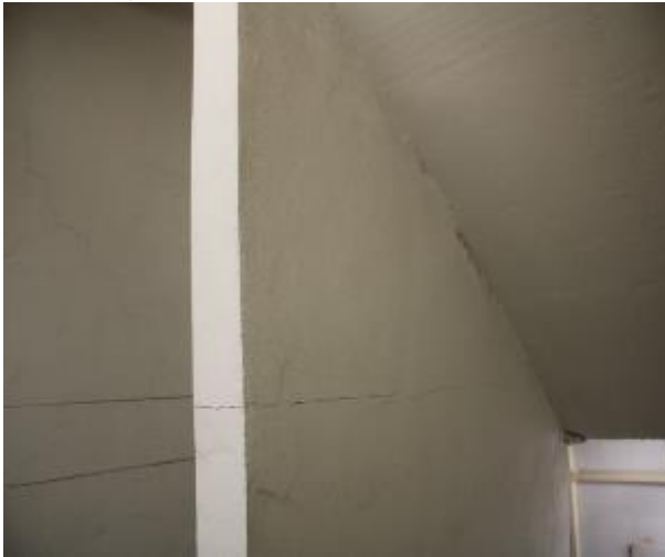
Figure 321 - Crack propagation through level 5 to basement B2 fire stairs internal wall
