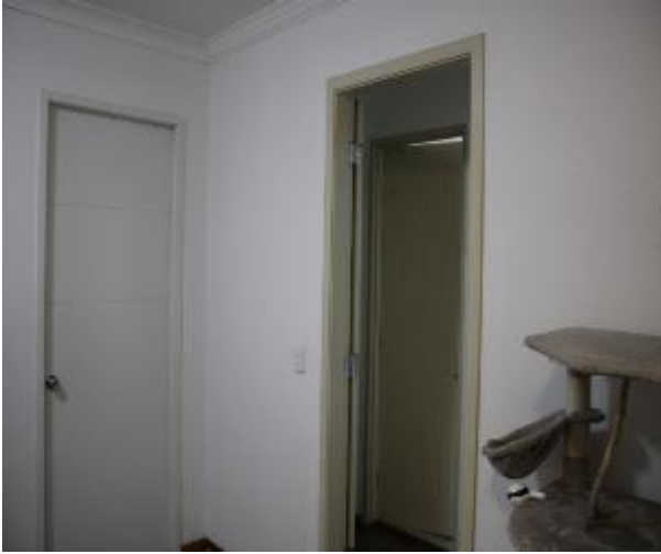
Figure 1272 - General condition of dining room internal wall
