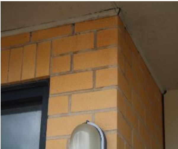
Figure 1400 - Crack propagation through external wall
