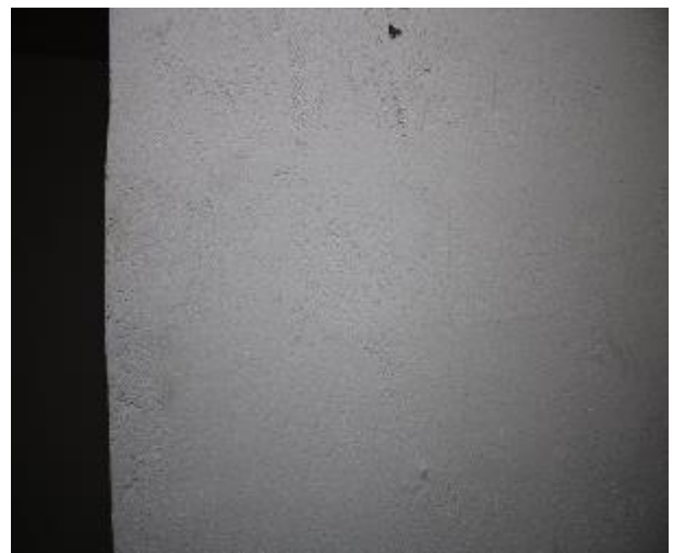
Figure 230 - Crack propagation through level 5 to basement B2 fire stairs internal wall
