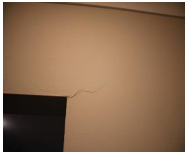
Figure 899 - Crack propagation through corridor internal wall
