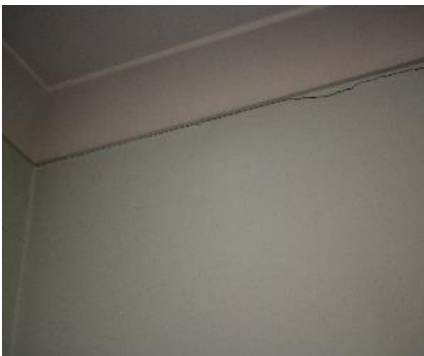
Figure 1198 - Crack propagation through study internal wall
