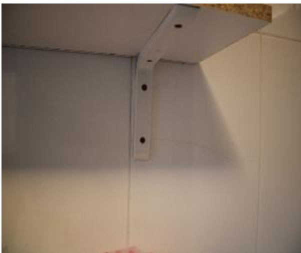
Figure 714 - Crack propagation through ensuite bathroom internal wall
