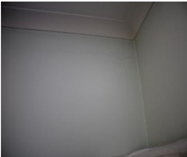
Figure 1196 - Crack propagation through study internal wall
