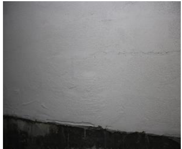
Figure 420 - Crack propagation through level 5 to basement B2 fire stairs internal wall
