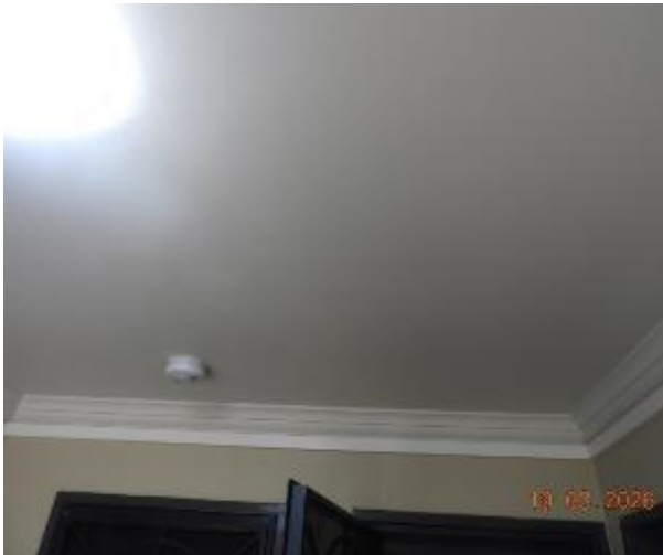
Figure 21 - General condition of level 1 common area ceiling
