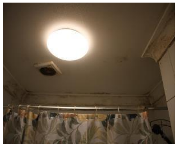
Figure 1385 - Water damage evident through ensuite bathroom ceiling
