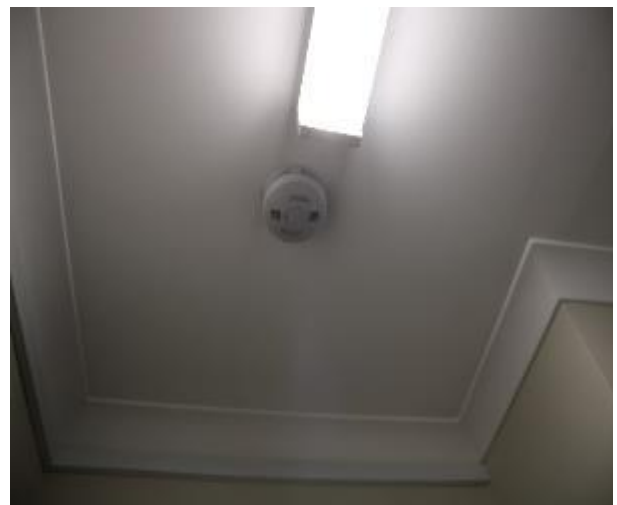
Figure 150 - General condition of level 5 common area ceiling
