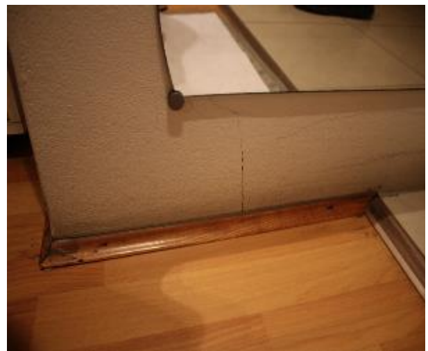
Figure 1085 - Crack propagation through lounge room internal wall
