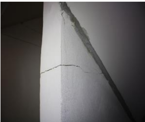
Figure 349 - Crack propagation through level 5 to basement B2 fire stairs internal wall
