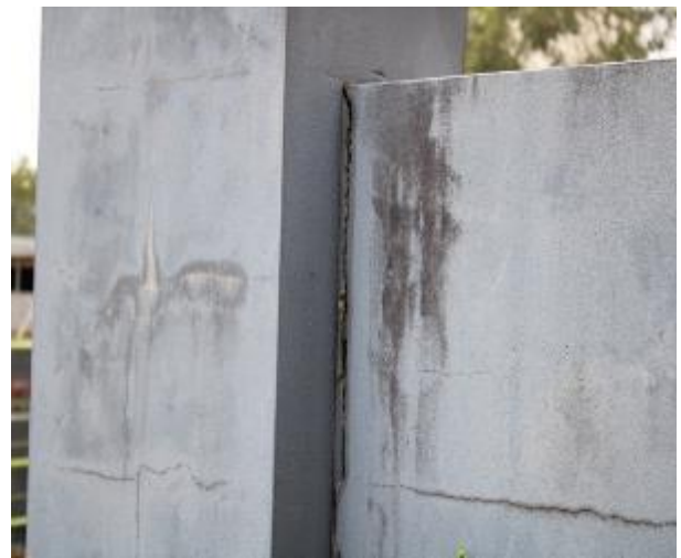
Figure 1583 - Crack propagation through external wall
