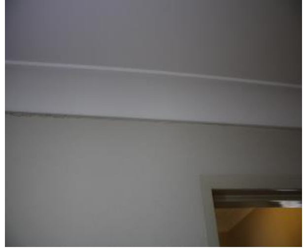
Figure 1485 - Crack propagation through bedroom 1 ceiling
