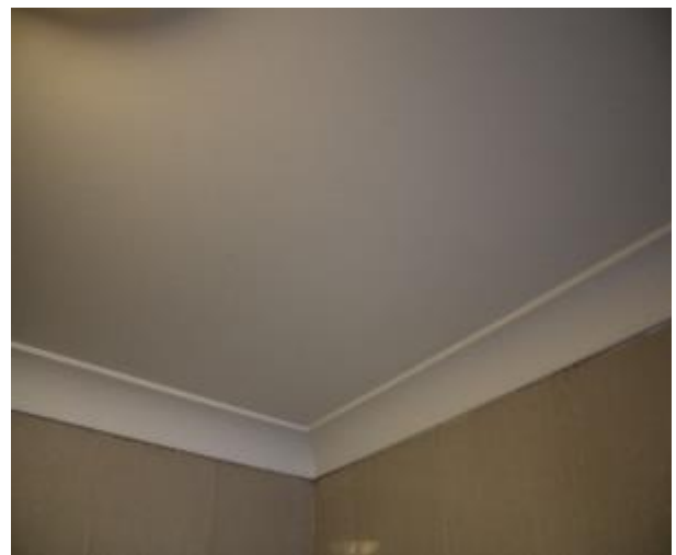
Figure 1193 - General condition of bathroom 1 ceiling
