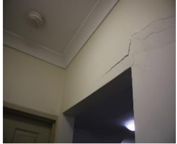
Figure 581 - Crack propagation through corridor internal wall
