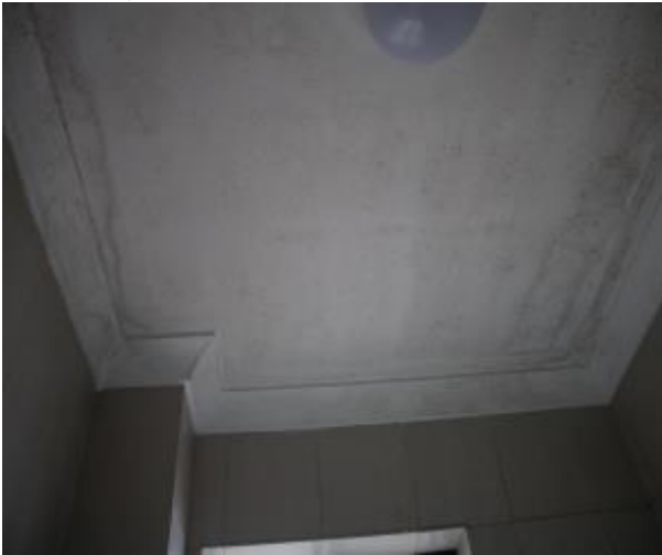
Figure 1356 - Water damage evident through bathroom 1 ceiling
