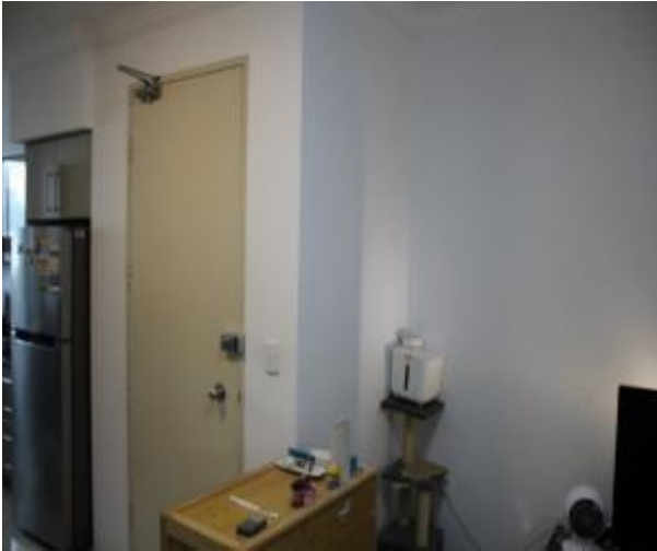
Figure 1274 - General condition of dining room internal wall
