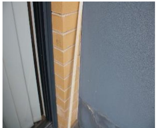
Figure 1317 - Crack propagation through external wall
