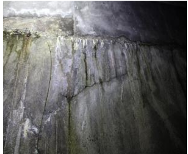
Figure 472 - Crack propagation and water damage through basement B2 fire stairs internal wall
