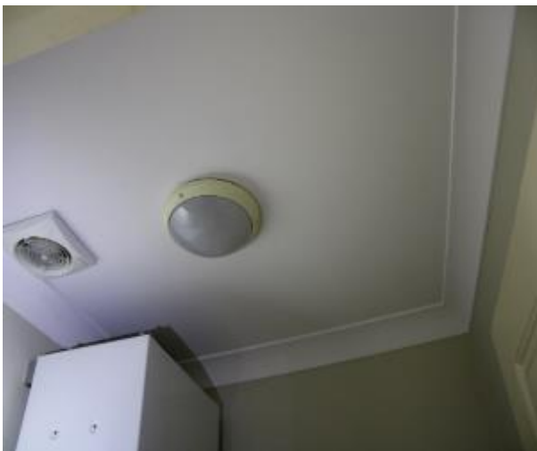
Figure 908 - General condition of laundry ceiling
