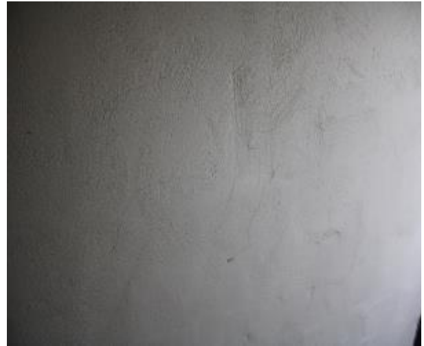
Figure 382 - Crack propagation through level 5 to basement B2 fire stairs internal wall
