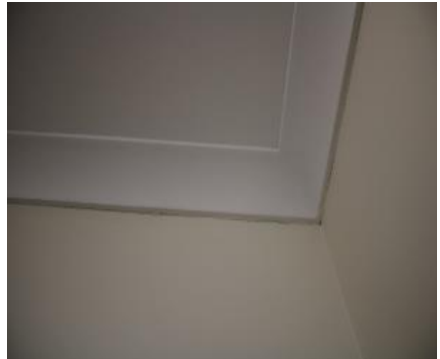
Figure 529 - Crack propagation through corridor ceiling
