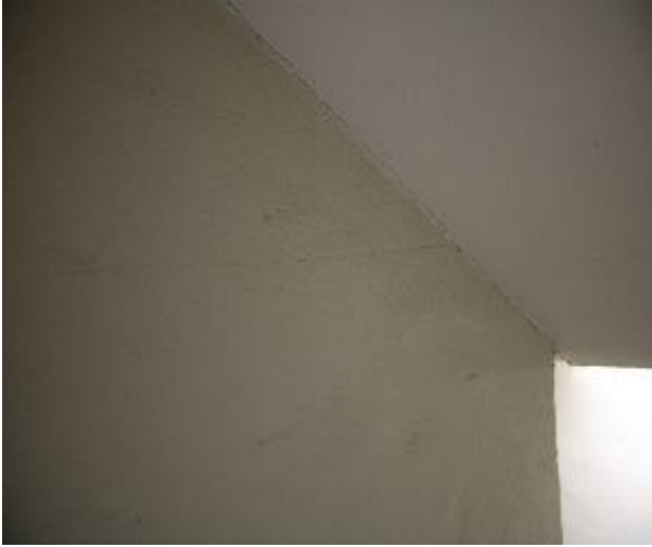
Figure 297 - Crack propagation through level 5 to basement B2 fire stairs internal wall
