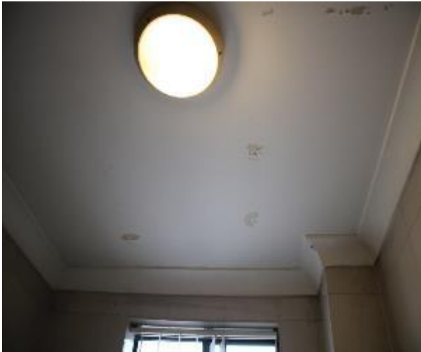
Figure 1544 - General condition of bathroom 1 ceiling
