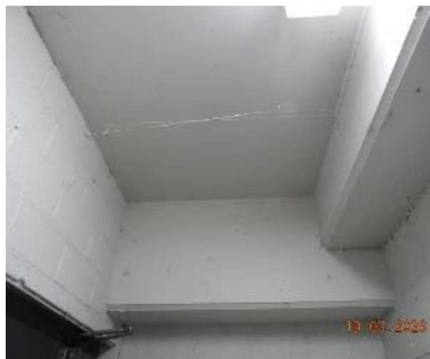
Figure 188 - General condition of B2 to Level 1 fire stairs underside slab
