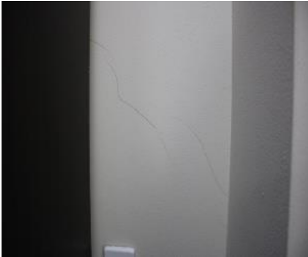
Figure 816 - Crack propagation through open kitchen/ lounge room internal wall
