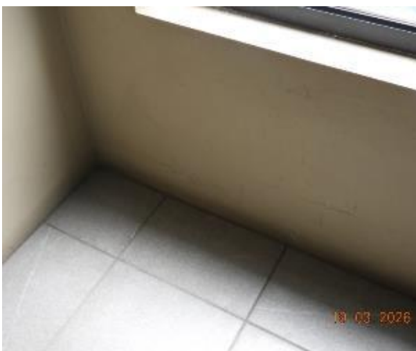
Figure 41 - Crack propagation through level 2 common area internal wall
