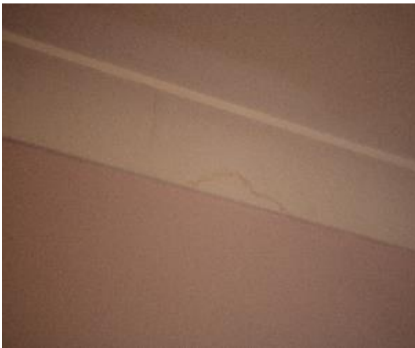
Figure 1142 - Crack propagation through bedroom 1 ceiling
