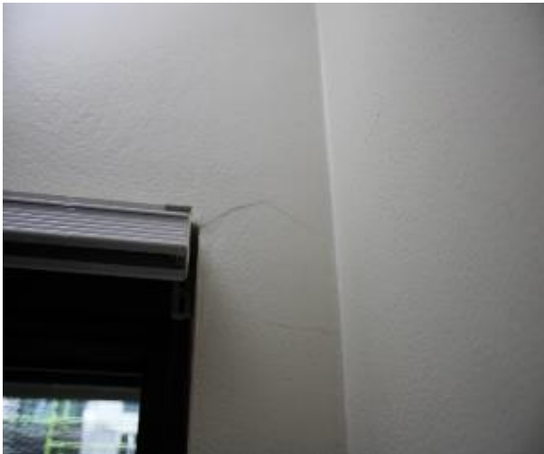
Figure 1100 - Crack propagation through lounge room internal wall
