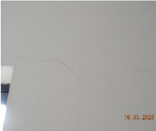
Figure 37 - Crack propagation through level 2 common area internal wall
