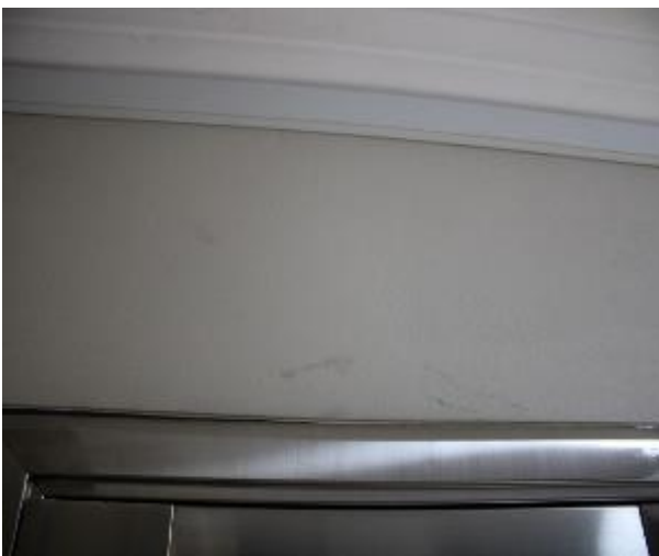
Figure 107 - Crack propagation through level 4 common area internal wall
