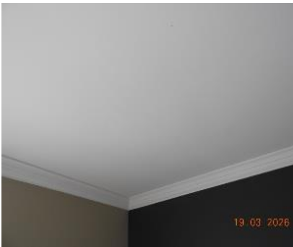
Figure 51 - General condition of level 2 common area ceiling
