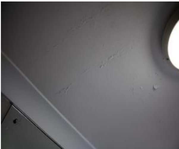
Figure 620 - Paint flaking through bathroom 1 ceiling
