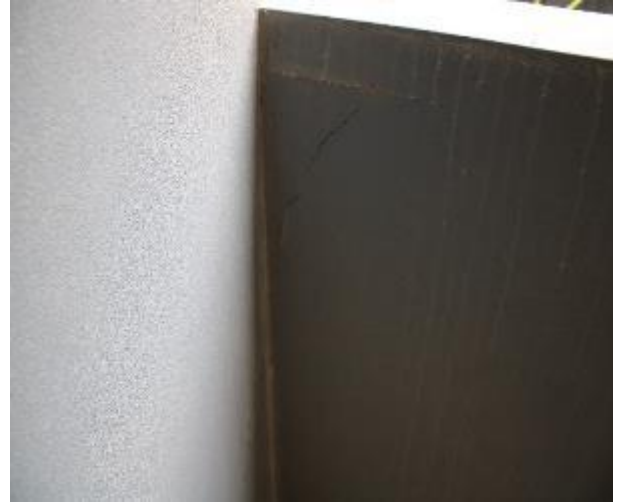
Figure 653 - Crack propagation through external wall
