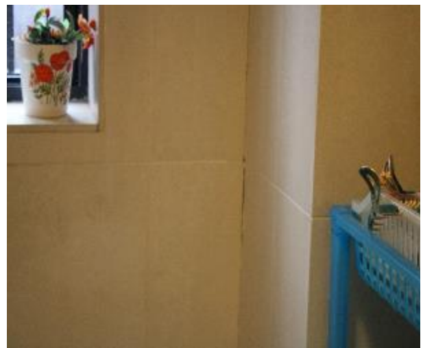
Figure 1034 - Crack propagation through bathroom 1 internal wall
