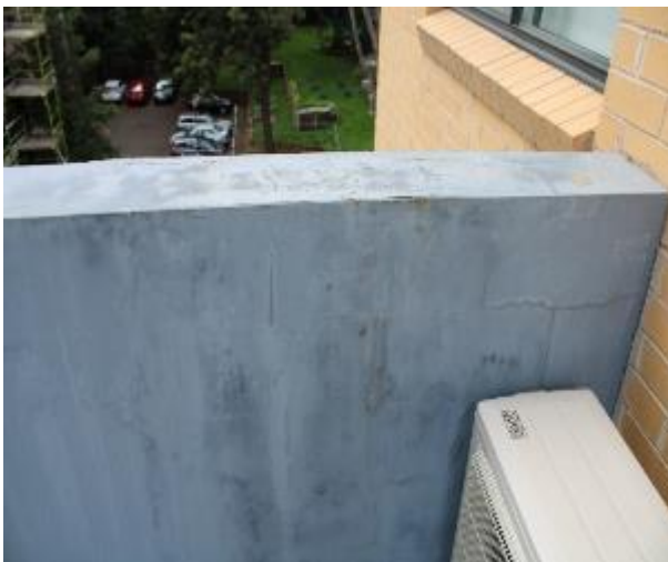
Figure 1304 - Crack propagation through external wall
