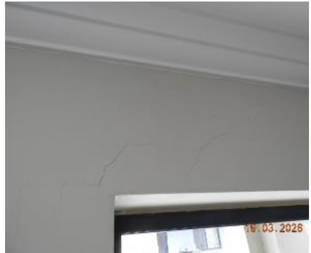
Figure 10 - Crack propagation through level 1 common area internal wall
