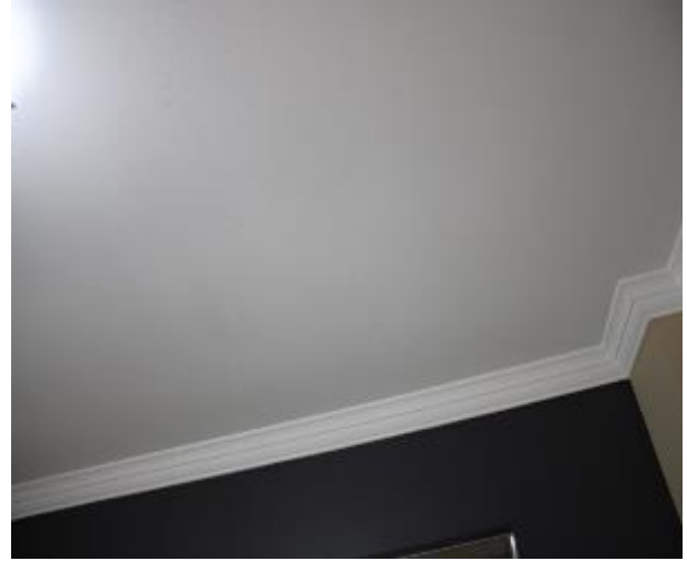
Figure 110 - General condition of level 4 common area ceiling
