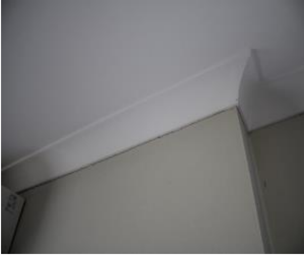
Figure 1490 - Crack propagation through bedroom 1 ceiling
