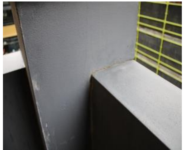
Figure 1239 - Crack propagation through external wall
