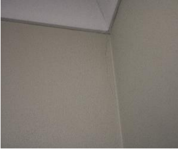
Figure 1466 - Crack propagation through corridor internal wall
