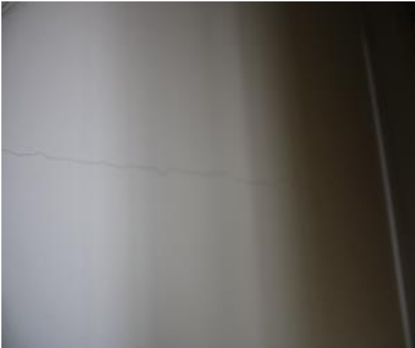
Figure 1442 - Crack propagation through laundry internal wall
