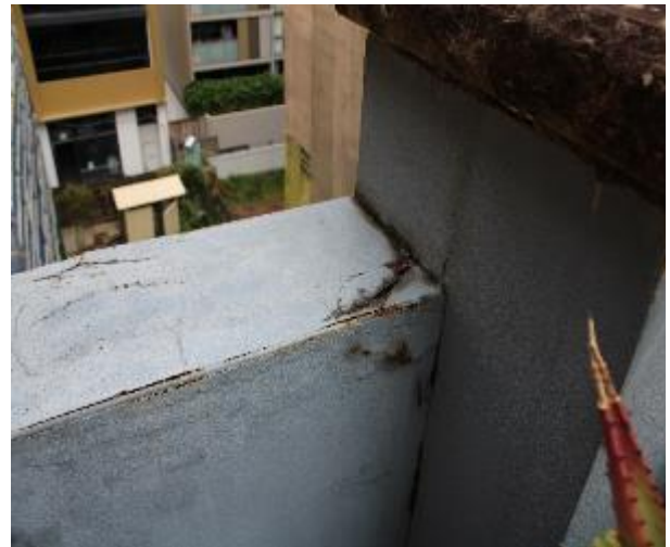
Figure 1589 - Crack propagation through external wall
