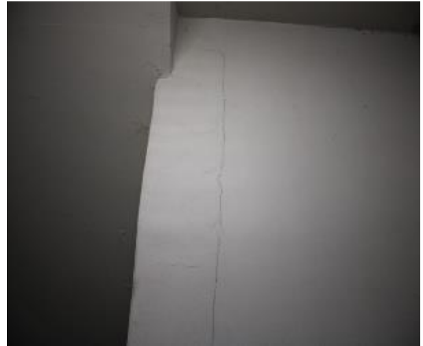
Figure 400 - Crack propagation through level 5 to basement B2 fire stairs internal wall
