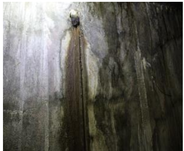
Figure 468 - Water damage evident through basement B2 fire stairs internal wall
