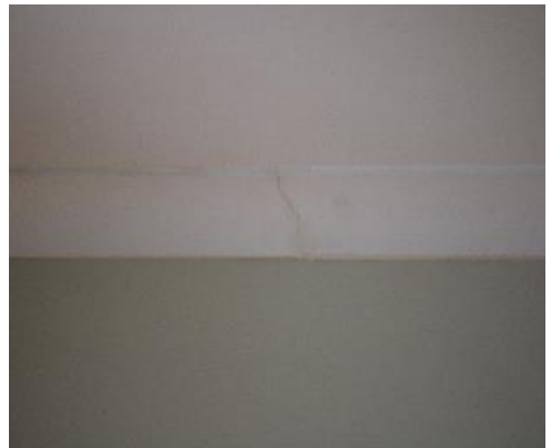
Figure 863 - Crack propagation through bedroom 1 ceiling
