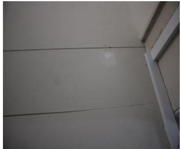
Figure 124 - Crack propagation through staircase to level 5 common area internal wall
