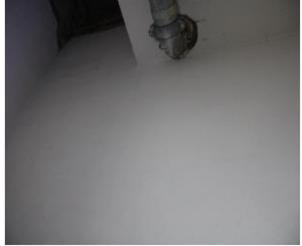
Figure 418 - Crack propagation through level 5 to basement B2 fire stairs internal wall
