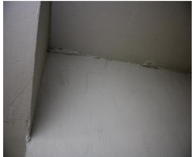
Figure 294 - Crack propagation through level 5 to basement B2 fire stairs internal wall
