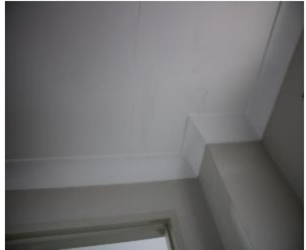
Figure 1443 - General condition of laundry ceiling
