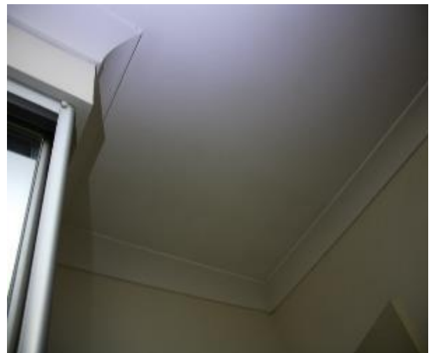
Figure 595 - General condition of bedroom 2 ceiling
