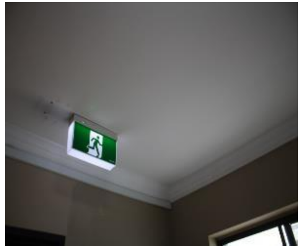
Figure 112 - General condition of level 4 common area ceiling
