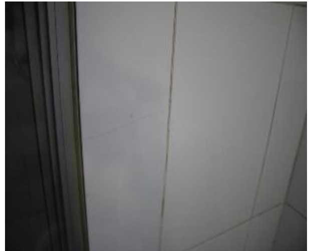
Figure 565 - Crack propagation through ensuite bathroom internal wall
