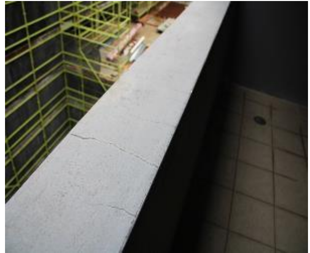
Figure 1243 - Crack propagation through external wall
