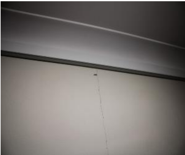
Figure 147 - Crack propagation through level 5 common area internal wall
