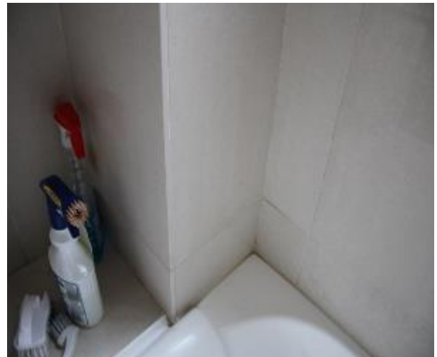
Figure 1347 - Crack propagation through bathroom 1 internal wall
