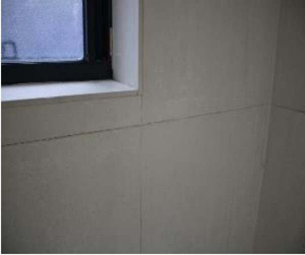
Figure 740 - Crack propagation through bathroom 1 internal wall
