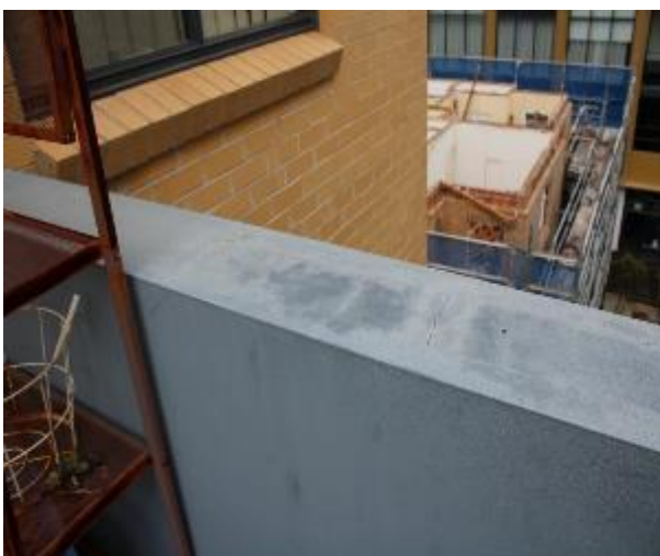
Figure 1590 - Crack propagation through external wall
