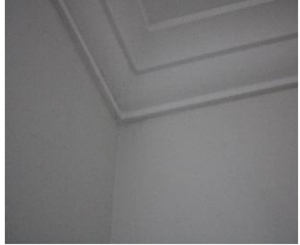
Figure 675 - Crack propagation through kitchen ceiling
