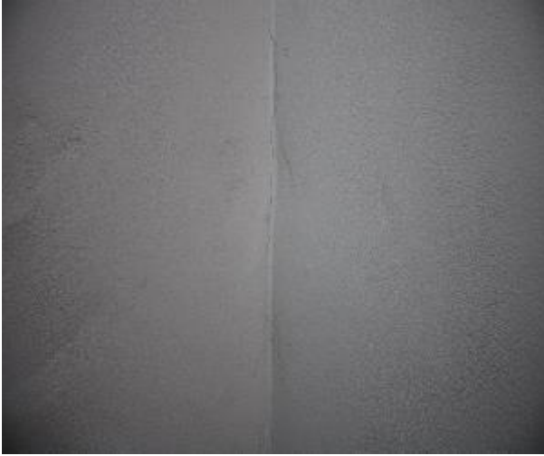
Figure 339 - Crack propagation through level 5 to basement B2 fire stairs internal wall
