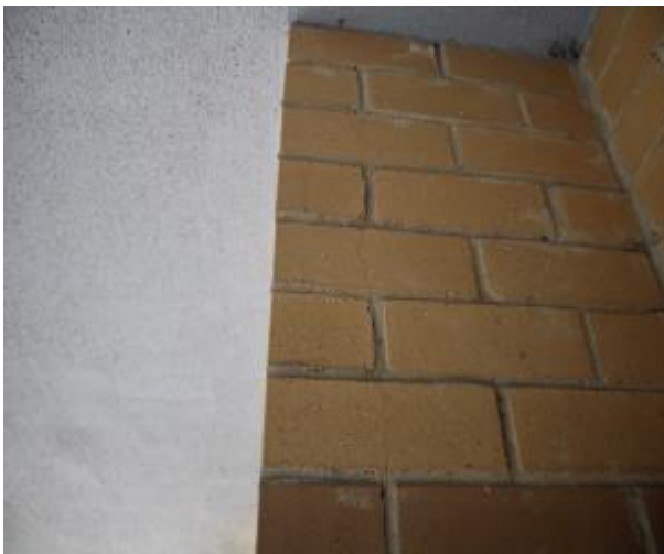
Figure 644 - Crack propagation through external wall
