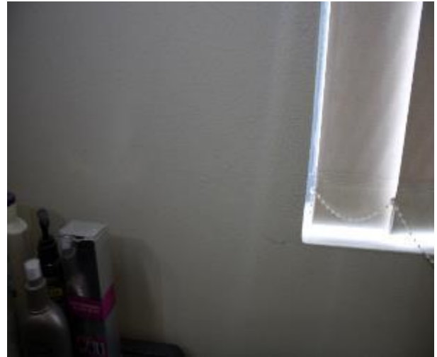
Figure 883 - Crack propagation through bedroom 2 internal wall
