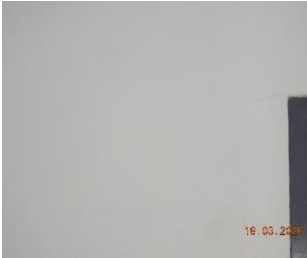
Figure 49 - Crack propagation through level 2 common area internal wall
