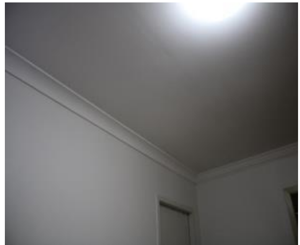
Figure 1277 - General condition of dining room ceiling
