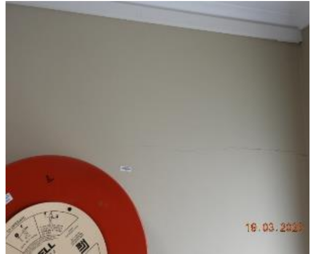
Figure 68 - Crack propagation through level 3 common area internal wall
