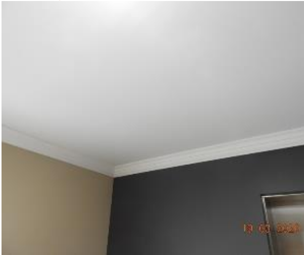
Figure 79 - General condition of level 3 common area ceiling
