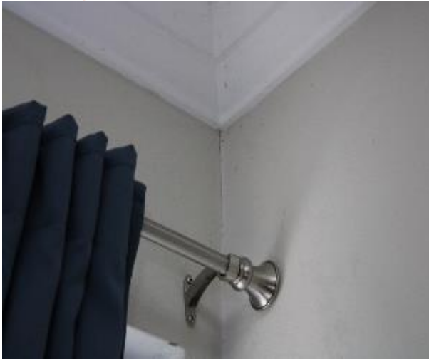
Figure 1454 - Crack propagation through lounge room internal wall
