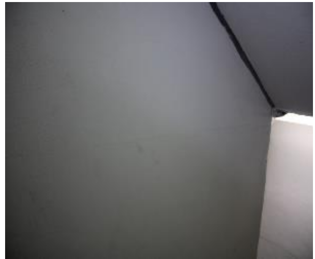
Figure 348 - Crack propagation through level 5 to basement B2 fire stairs internal wall
