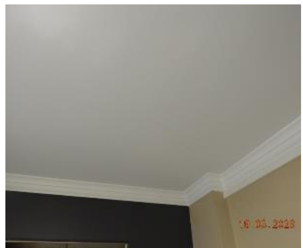
Figure 78 - General condition of level 3 common area ceiling
