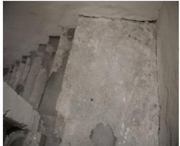
Figure 306 - General condition of level 5 to basement B2 fire stairs concrete floor
