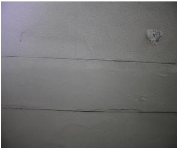
Figure 257 - Crack propagation through level 5 to basement B2 fire stairs internal wall
