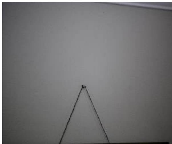
Figure 1449 - Crack propagation through lounge room internal wall
