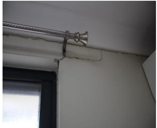
Figure 1475 - Crack propagation through bedroom 1 internal wall
