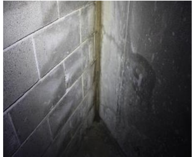
Figure 460 - Water damage evident through basement B2 fire stairs internal wall
