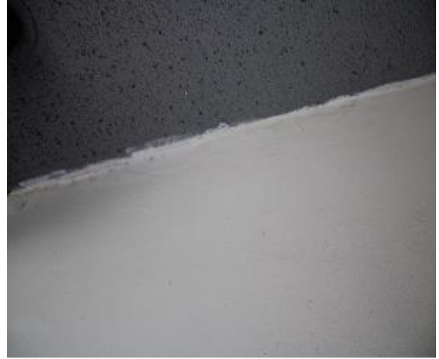
Figure 783 - Crack propagation through external wall
