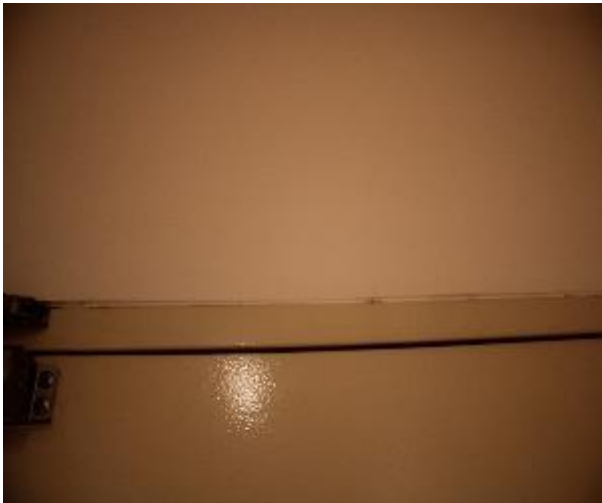
Figure 1088 - Crack propagation through lounge room internal wall
