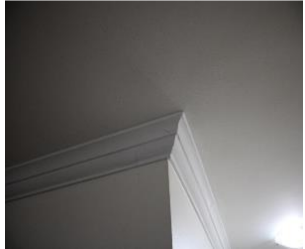
Figure 517 - Crack propagation through open kitchen/ lounge room ceiling
