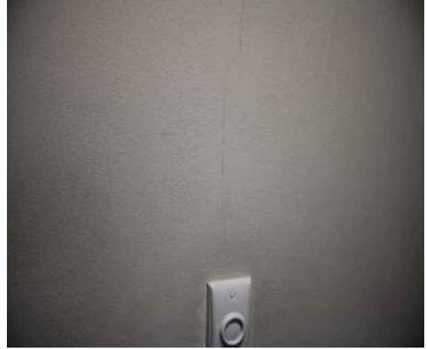
Figure 146 - Crack propagation through level 5 common area internal wall
