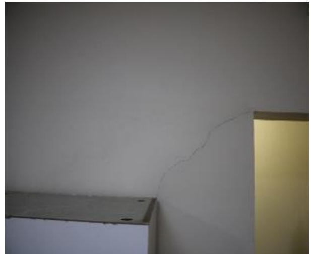
Figure 499 - Crack propagation through open kitchen/ lounge room internal wall
