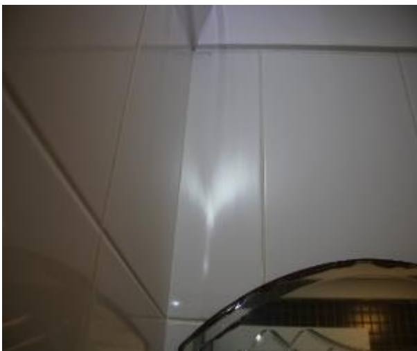
Figure 720 - Crack propagation through ensuite bathroom internal wall
