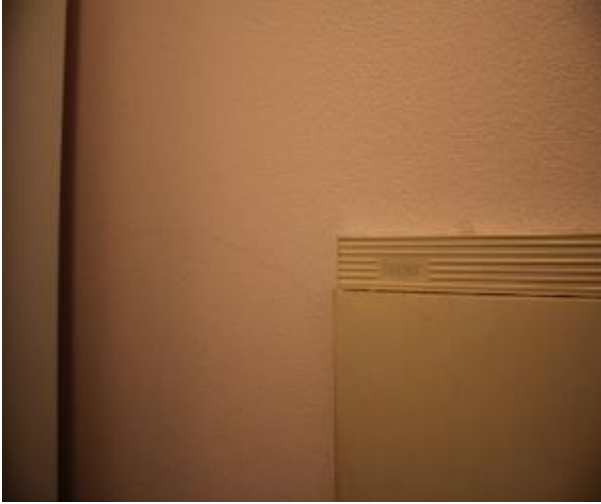
Figure 1122 - Crack propagation through bedroom 1 internal wall
