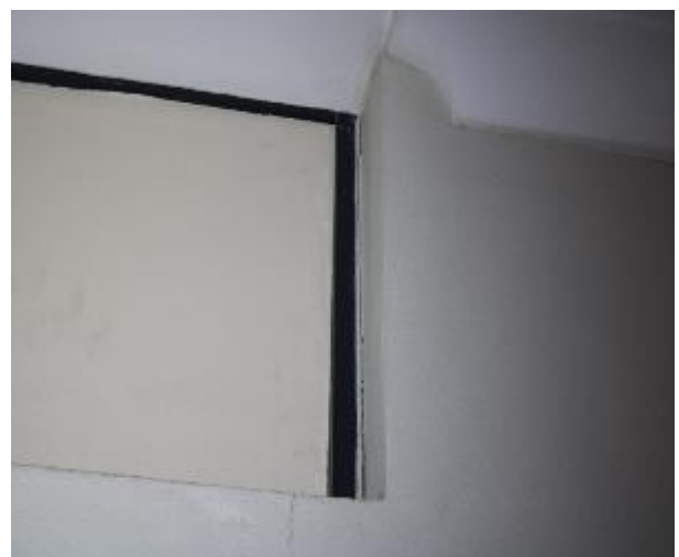
Figure 1549 - Crack propagation through bedroom 2 internal wall
