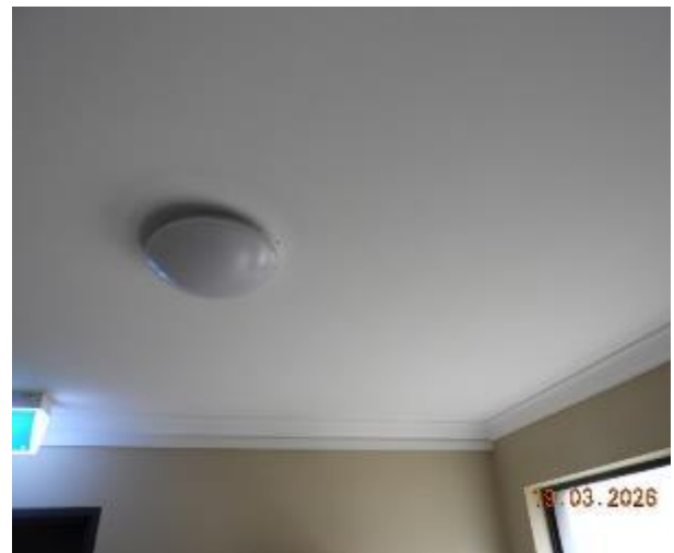
Figure 52 - General condition of level 2 common area ceiling
