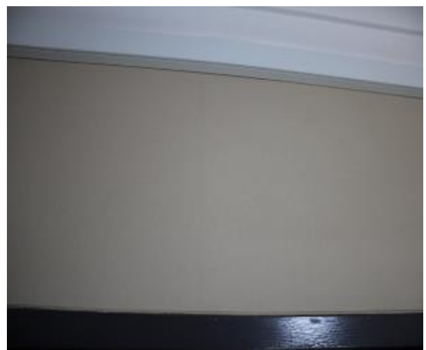
Figure 90 - Crack propagation through level 4 common area internal wall
