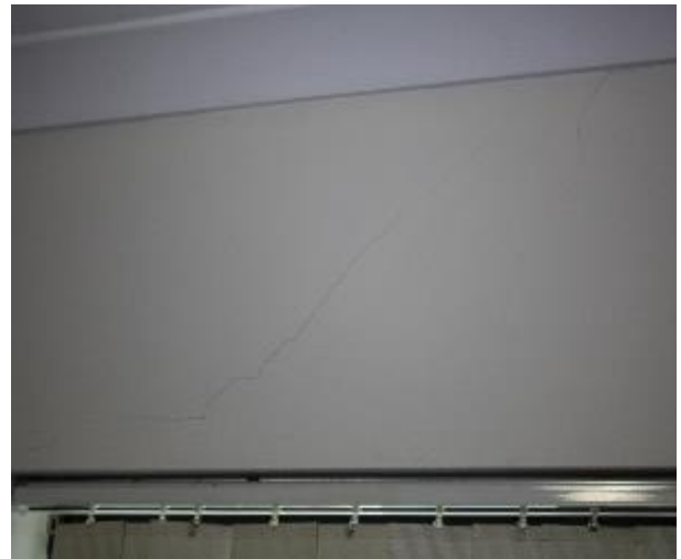
Figure 589 - Crack propagation through bedroom 2 internal wall
