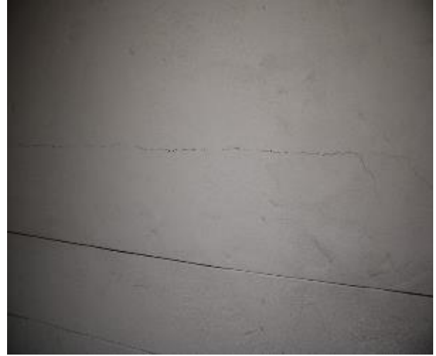
Figure 370 - Crack propagation through level 5 to basement B2 fire stairs internal wall
