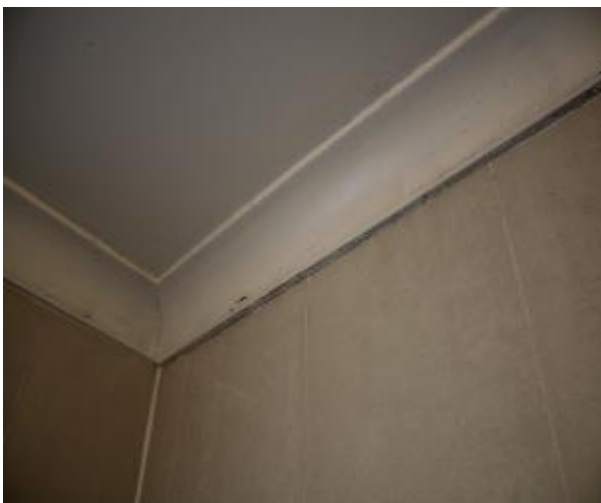
Figure 850 - Crack propagation through bathroom 1 ceiling
