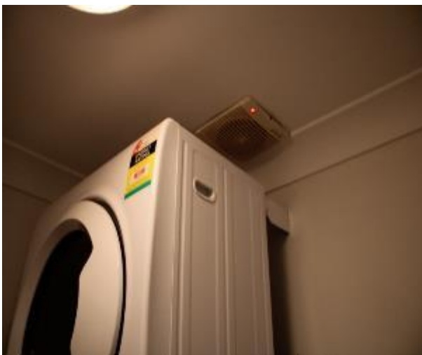
Figure 696 - General condition of laundry ceiling
