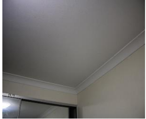
Figure 557 - General condition of bedroom 1 ceiling
