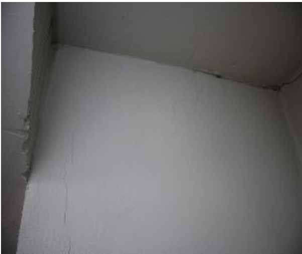
Figure 341 - Crack propagation through level 5 to basement B2 fire stairs internal wall
