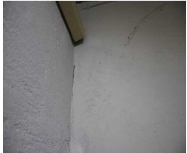
Figure 238 - Crack propagation through level 5 to basement B2 fire stairs internal wall
