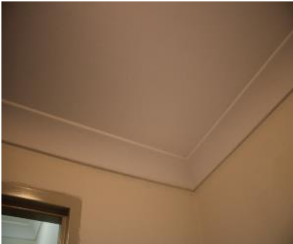
Figure 540 - General condition of laundry ceiling
