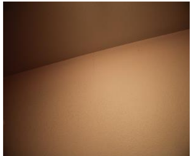
Figure 1121 - Crack propagation through bedroom 1 internal wall
