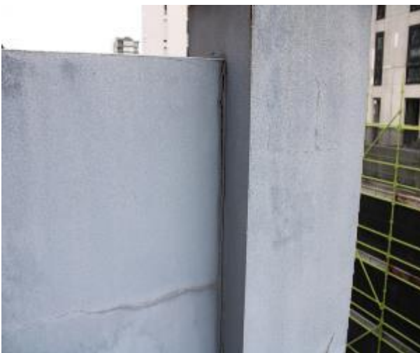
Figure 1312 - Crack propagation through external wall
