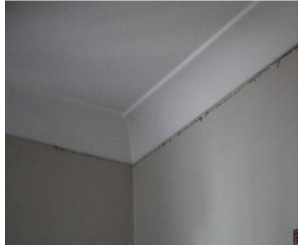
Figure 1487 - Crack propagation through bedroom 1 ceiling
