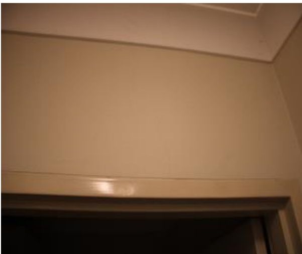
Figure 902 - Crack propagation through corridor internal wall
