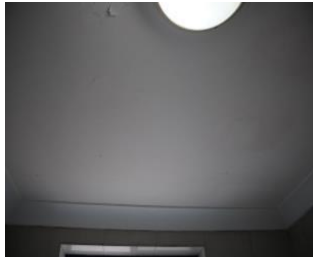
Figure 619 - General condition of bathroom 1 ceiling
