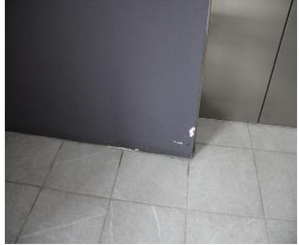
Figure 92 - Paint flaking through level 4 common area internal wall
