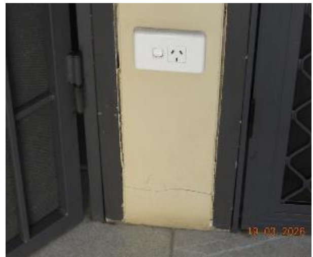
Figure 46 - Crack propagation through level 2 common area internal wall
