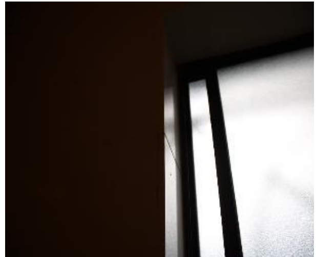
Figure 1038 - Crack propagation through bathroom 1 internal wall
