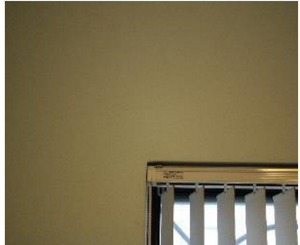
Figure 1171 - Crack propagation through bedroom 2 internal wall
