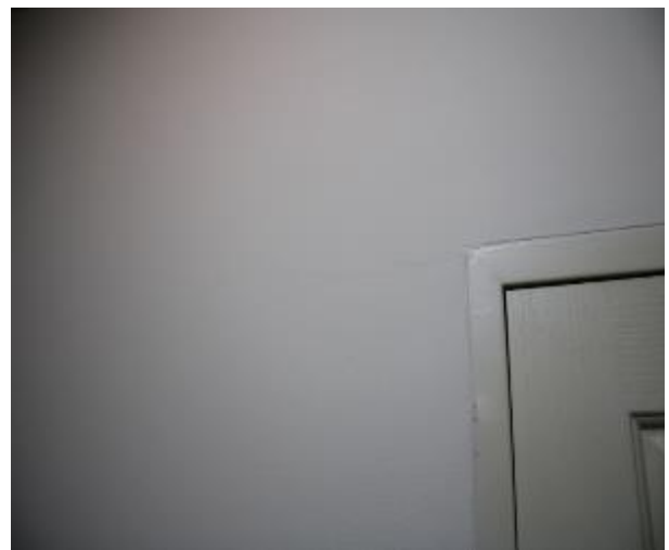
Figure 809 - Crack propagation through open kitchen/ lounge room internal wall
