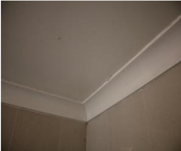
Figure 852 - General condition of bathroom 1 ceiling
