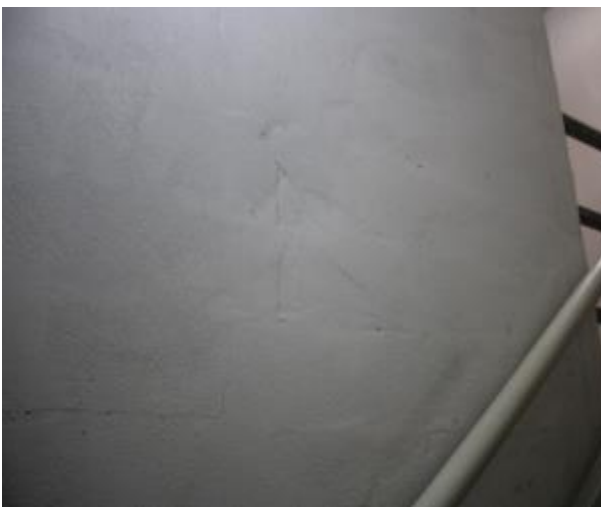
Figure 421 - Crack propagation through level 5 to basement B2 fire stairs internal wall
