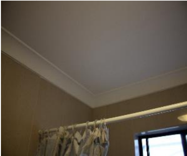
Figure 1047 - General condition of bathroom 1 ceiling
