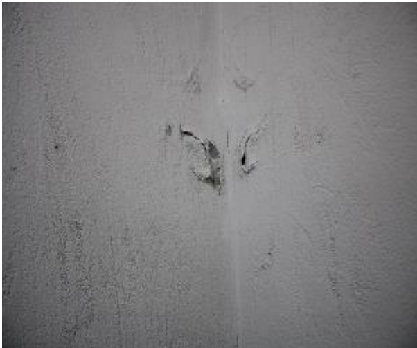
Figure 227 - Paint flaking through level 5 to basement B2 fire stairs internal wall
