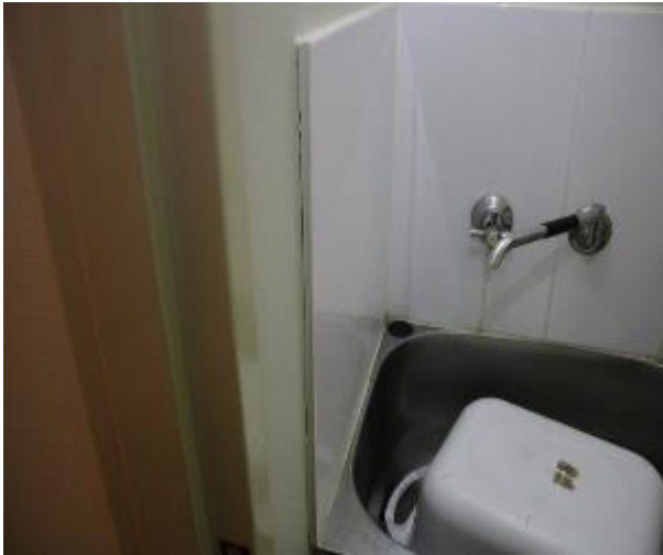
Figure 906 - Crack propagation through laundry internal wall
