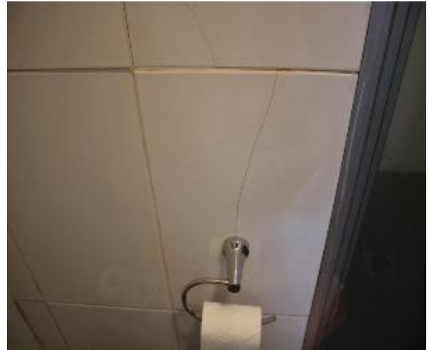
Figure 711 - Crack propagation through ensuite bathroom internal wall
