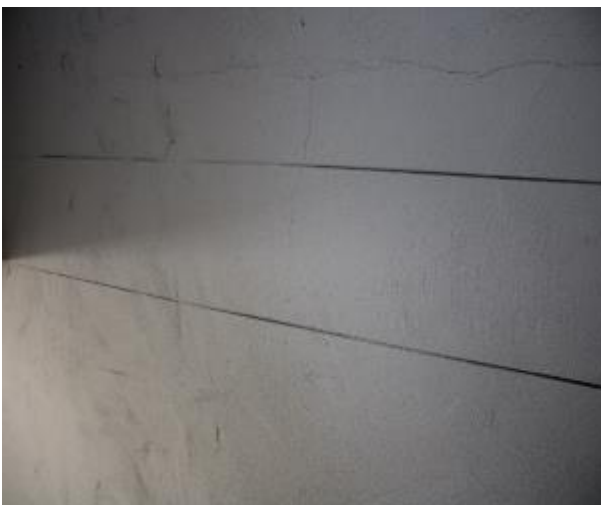
Figure 265 - Crack propagation through level 5 to basement B2 fire stairs internal wall
