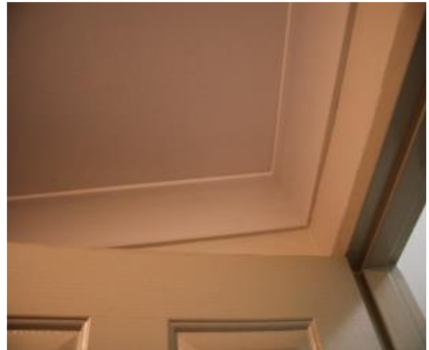
Figure 541 - General condition of laundry ceiling
