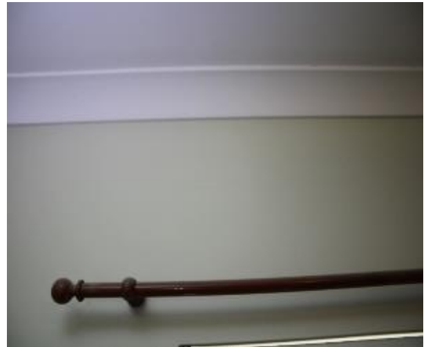
Figure 885 - Crack propagation through bedroom 2 internal wall
