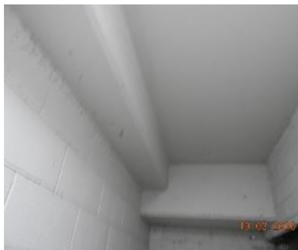
Figure 190 - General condition of B2 to Level 1 fire stairs underside slab
