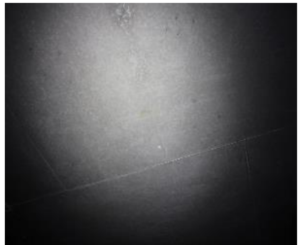
Figure 450 - Crack propagation through basement B2 fire stairs underside slab
