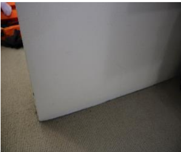
Figure 506 - Crack propagation through open kitchen/ lounge room internal wall
