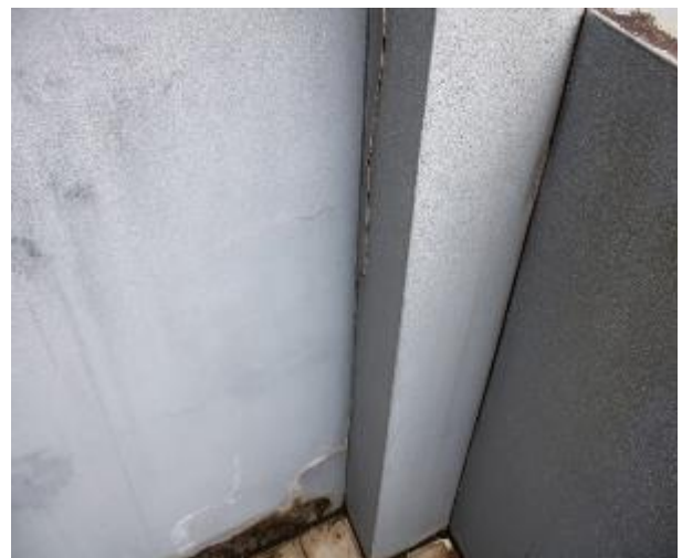
Figure 1313 - Crack propagation through external wall
