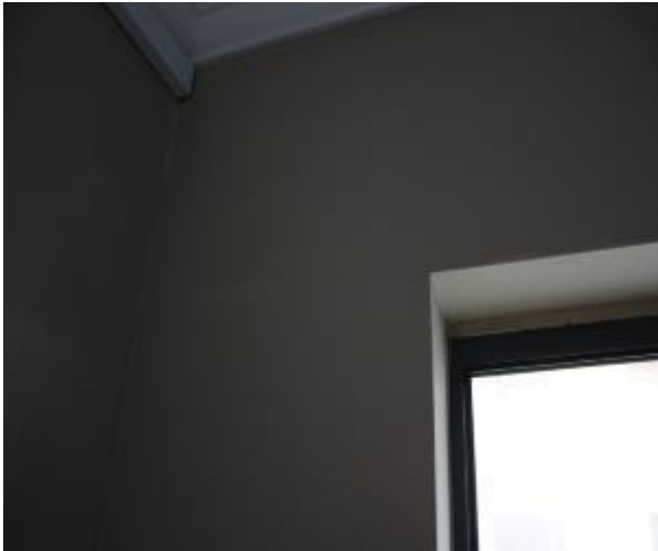
Figure 97 - Crack propagation through level 4 common area internal wall
