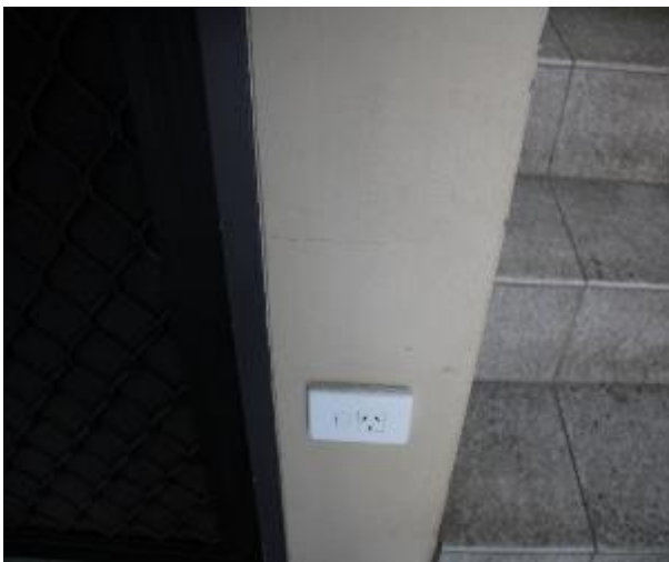
Figure 87 - Crack propagation through level 4 common area internal wall
