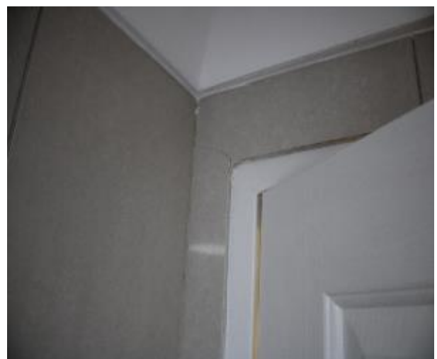
Figure 751 - Crack propagation through bathroom 1 internal wall
