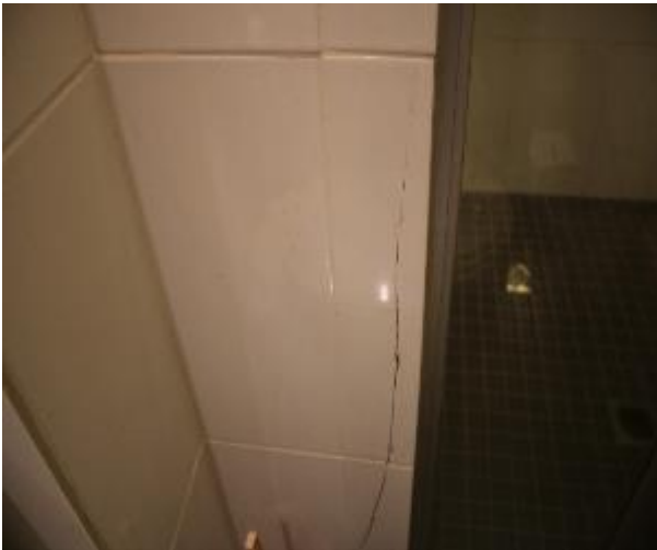
Figure 1148 - Crack propagation through ensuite bathroom internal wall
