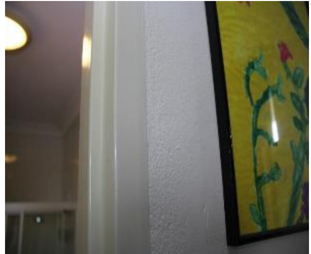
Figure 1479 - Crack propagation through bedroom 1 internal wall
