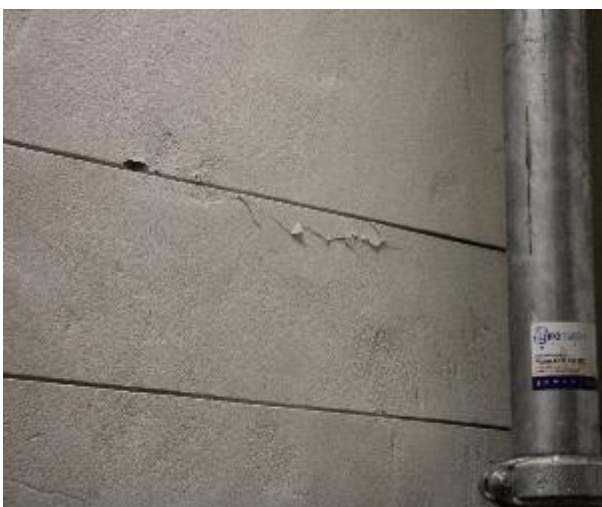
Figure 313 - Crack propagation through level 5 to basement B2 fire stairs internal wall
