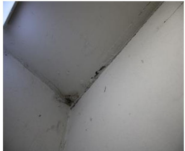
Figure 432 - Crack propagation through level 5 to basement B2 fire stairs underside stairs
