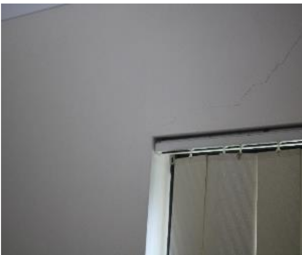
Figure 590 - Crack propagation through bedroom 2 internal wall
