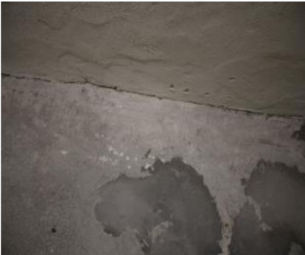
Figure 305 - Crack propagation through level 5 to basement B2 fire stairs concrete floor
