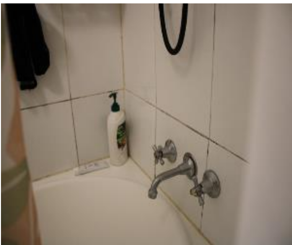
Figure 1378 - Crack propagation through ensuite bathroom internal wall
