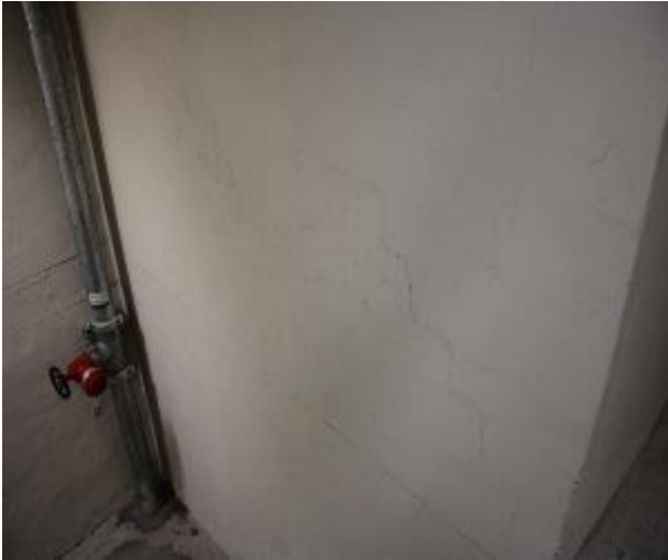
Figure 299 - Crack propagation through level 5 to basement B2 fire stairs internal wall
