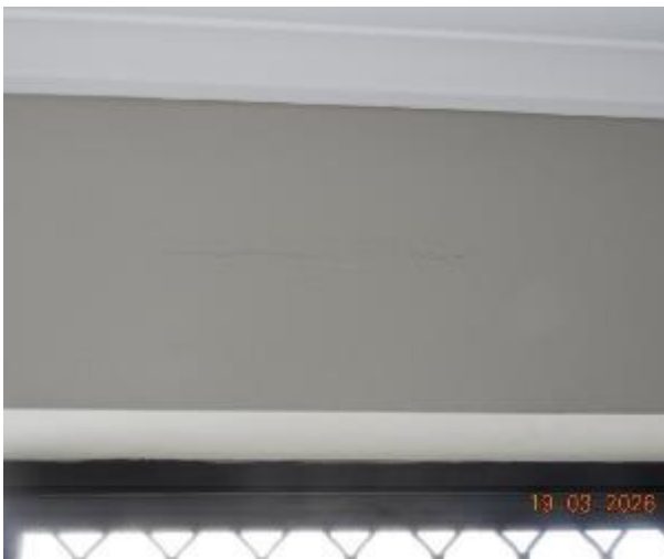
Figure 39 - Crack propagation through level 2 common area internal wall
