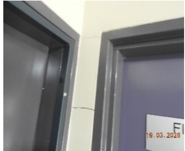
Figure 20 - Crack propagation through level 1 common area internal wall
