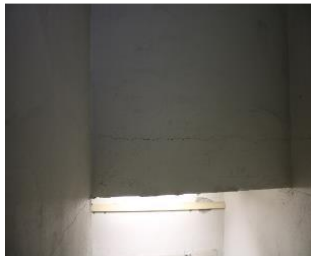
Figure 266 - Crack propagation through level 5 to basement B2 fire stairs internal wall
