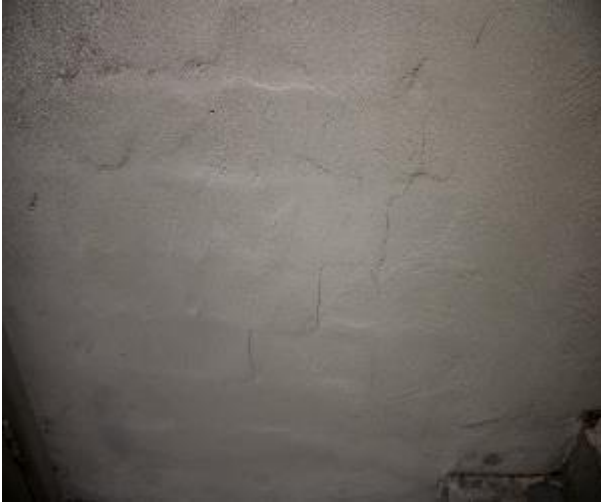
Figure 285 - Crack propagation through level 5 to basement B2 fire stairs internal wall
