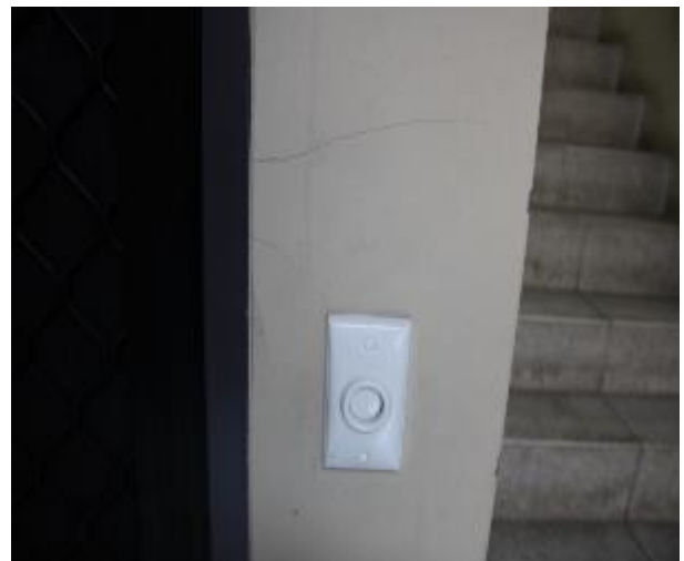
Figure 88 - Crack propagation through level 4 common area internal wall
