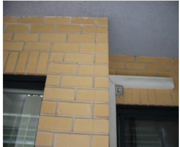
Figure 943 - Crack propagation through external wall
