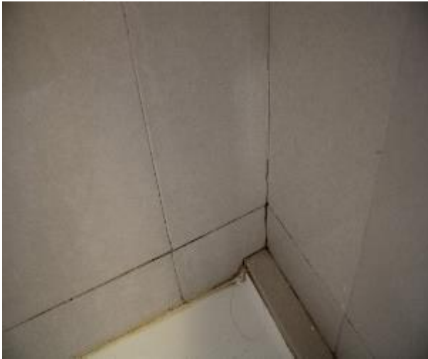
Figure 1035 - Crack propagation through bathroom 1 internal wall
