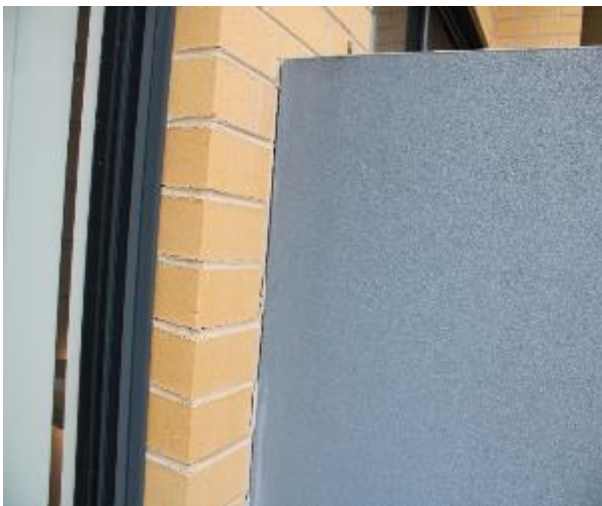
Figure 1316 - Crack propagation through external wall
