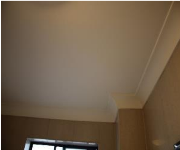
Figure 1194 - General condition of bathroom 1 ceiling
