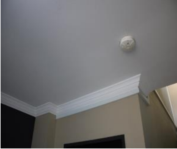
Figure 109 - General condition of level 4 common area ceiling
