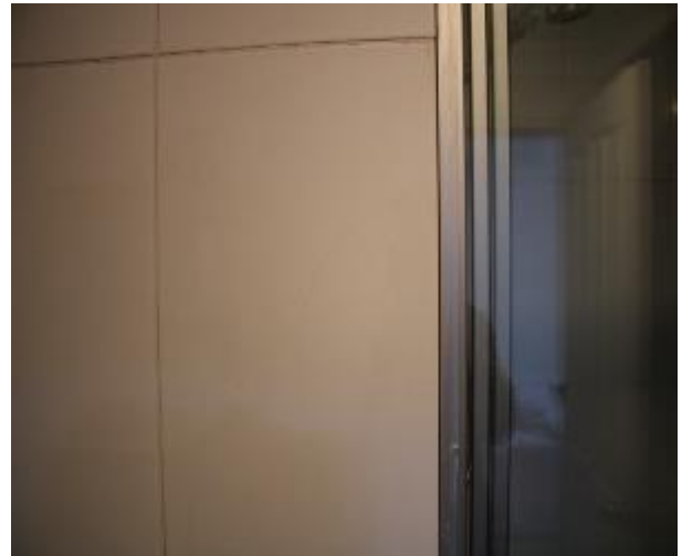
Figure 713 - Crack propagation through ensuite bathroom internal wall
