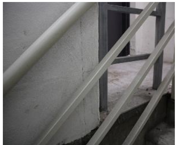
Figure 422 - Crack propagation through level 5 to basement B2 fire stairs internal wall
