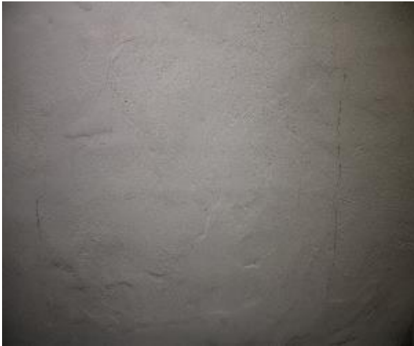
Figure 333 - Crack propagation through level 5 to basement B2 fire stairs internal wall
