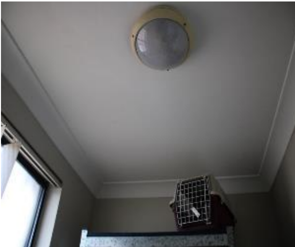
Figure 1444 - General condition of laundry ceiling
