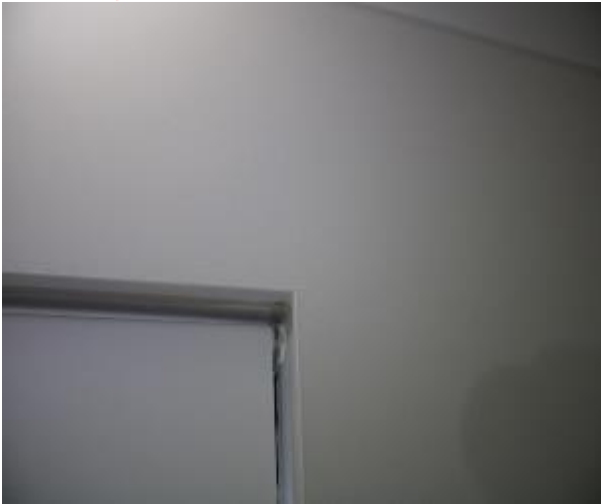
Figure 758 - Crack propagation through bedroom 3 internal wall
