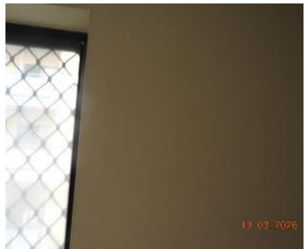
Figure 60 - Crack propagation through level 3 common area internal wall
