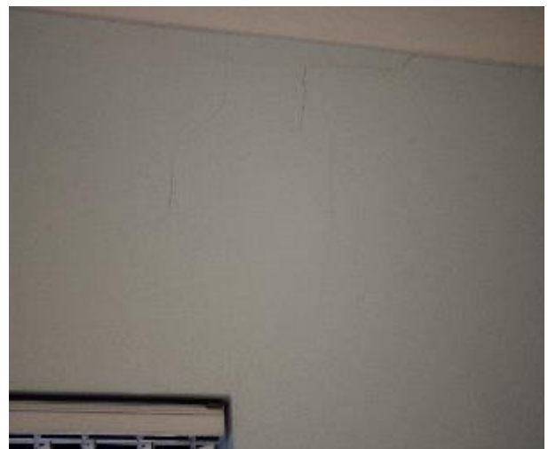
Figure 1169 - Crack propagation through bedroom 2 internal wall
