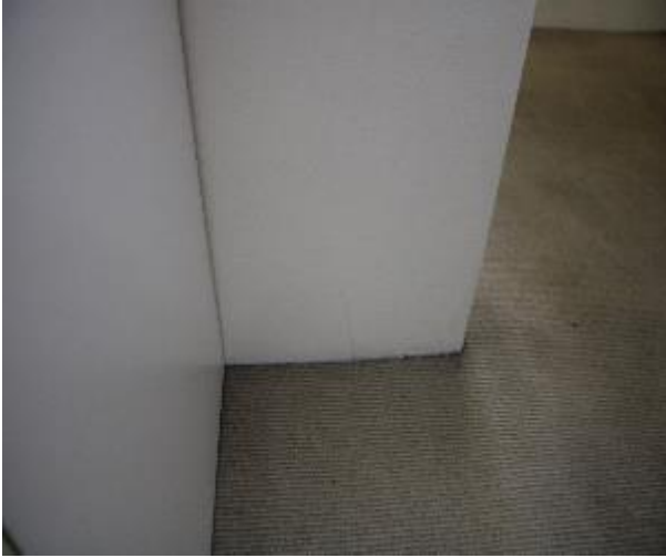
Figure 502 - Crack propagation through open kitchen/ lounge room internal wall
