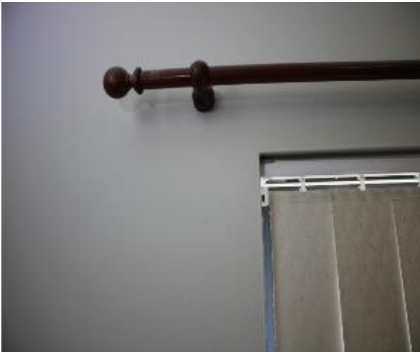
Figure 884 - Crack propagation through bedroom 2 internal wall
