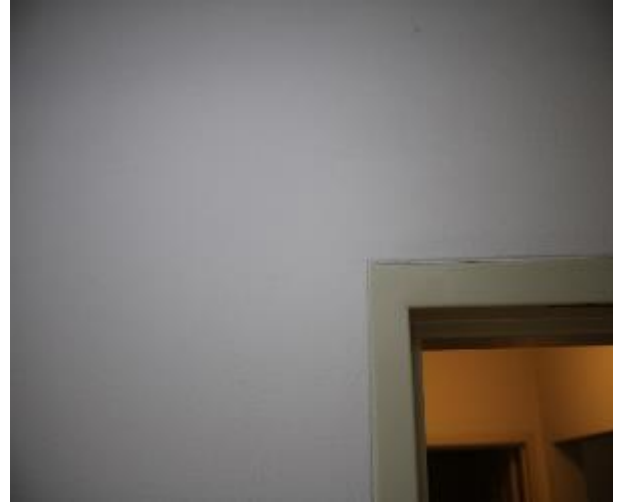
Figure 919 - Crack propagation through bedroom 3 internal wall
