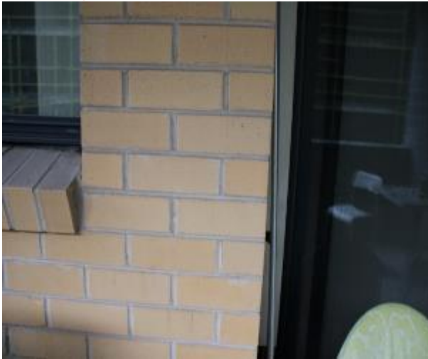
Figure 942 - Crack propagation through external wall
