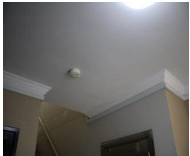
Figure 108 - General condition of level 4 common area ceiling
