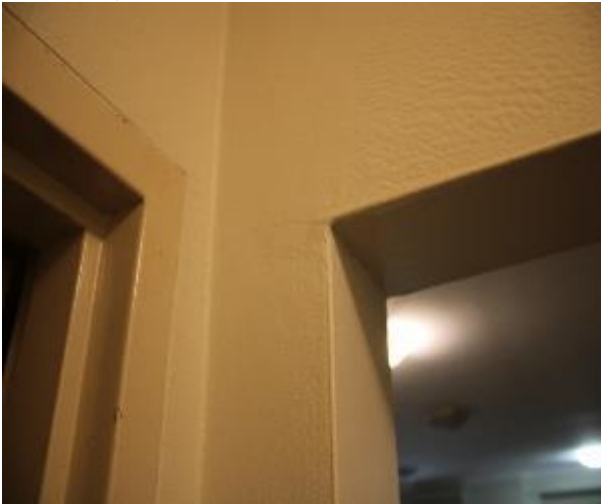
Figure 900 - Crack propagation through corridor internal wall
