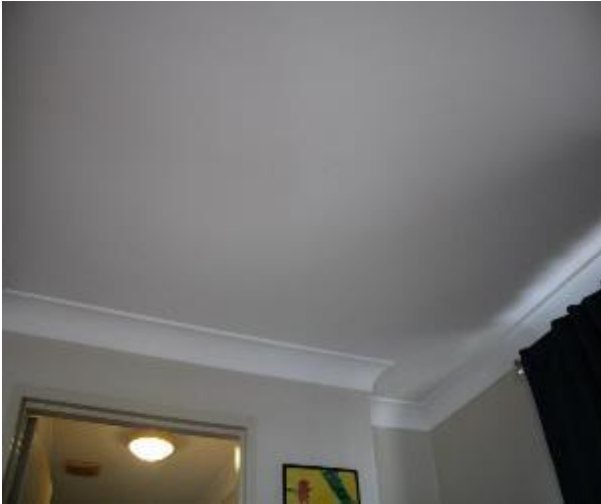
Figure 1492 - General condition of bedroom 1 ceiling
