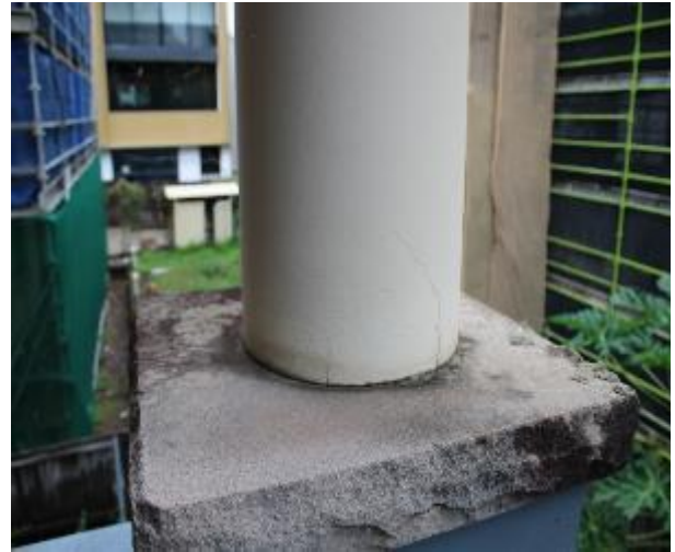
Figure 789 - Crack propagation through external wall
