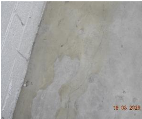
Figure 193 - Crack propagation through B2 to Level 1 fire stairs pavement slab
