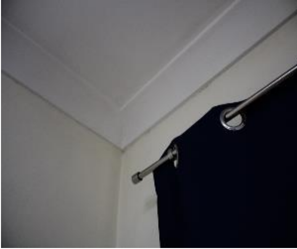
Figure 556 - Crack propagation through bedroom 1 ceiling
