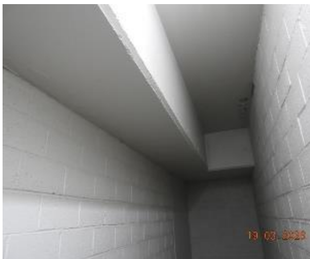
Figure 211 - General condition of B2 to Level 1 fire stairs underside slab
