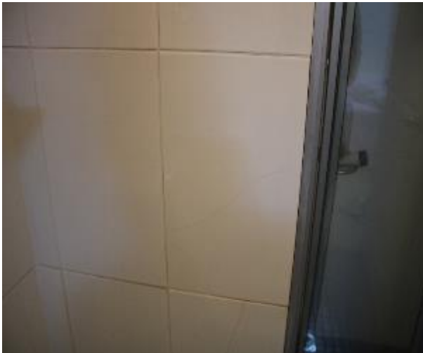
Figure 712 - Crack propagation through ensuite bathroom internal wall
