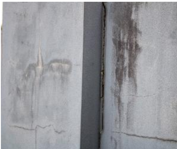
Figure 1582 - Crack propagation through external wall
