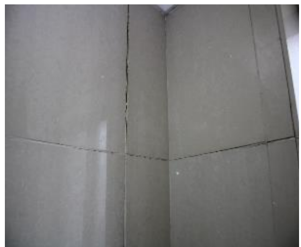
Figure 609 - Crack propagation through bathroom 1 internal wall
