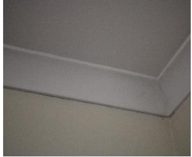
Figure 599 - Crack propagation through bedroom 2 ceiling
