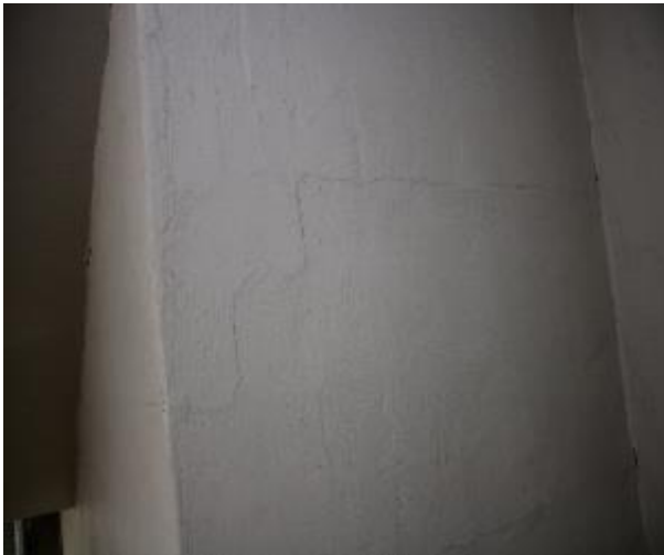
Figure 293 - Crack propagation through level 5 to basement B2 fire stairs internal wall
