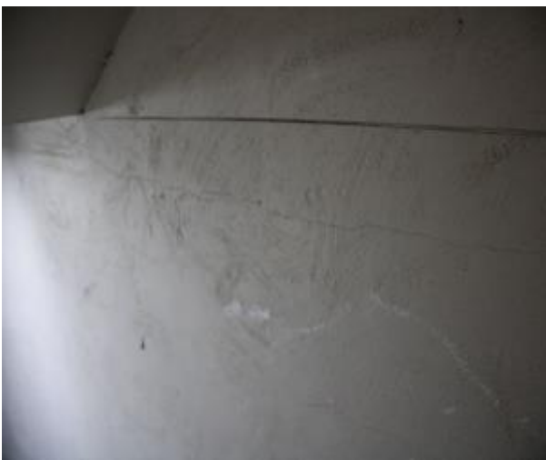
Figure 379 - Crack propagation through level 5 to basement B2 fire stairs internal wall
