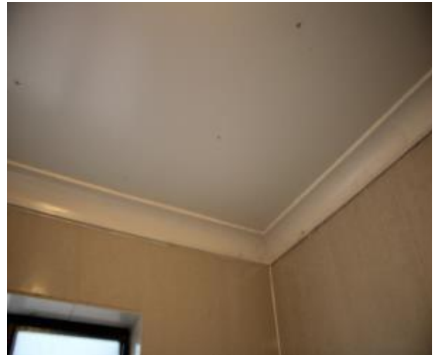
Figure 849 - General condition of bathroom 1 ceiling
