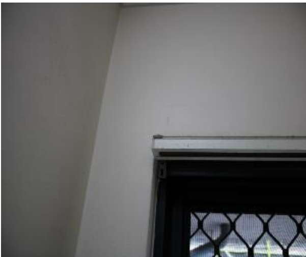
Figure 494 - Crack propagation through open kitchen/ lounge room internal wall
