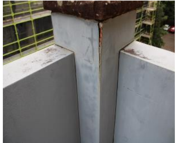
Figure 1303 - Crack propagation through external wall
