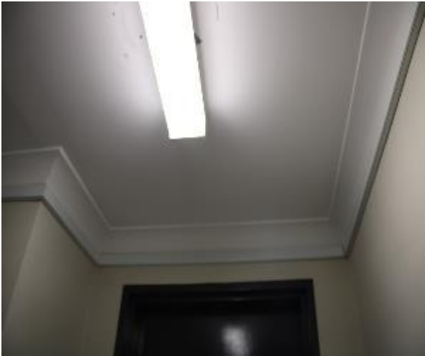
Figure 151 - General condition of level 5 common area ceiling
