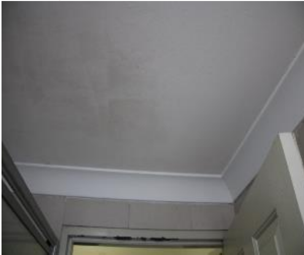
Figure 616 - General condition of bathroom 1 ceiling
