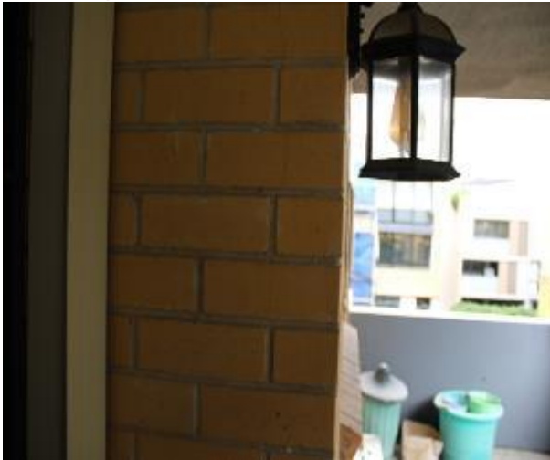
Figure 1065 - Crack propagation through external wall
