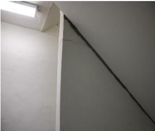
Figure 347 - Crack propagation through level 5 to basement B2 fire stairs internal wall
