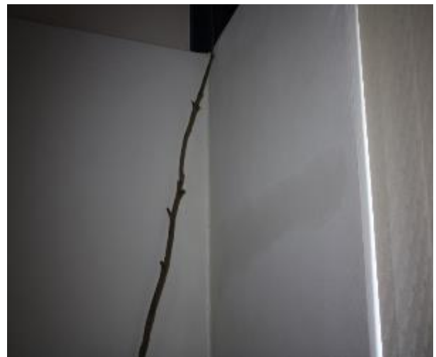
Figure 1553 - Crack propagation through bedroom 2 internal wall
