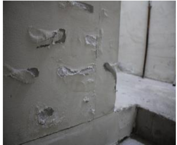
Figure 256 - Crack propagation and paint flaking through level 5 to basement B2 fire stairs internal wall
