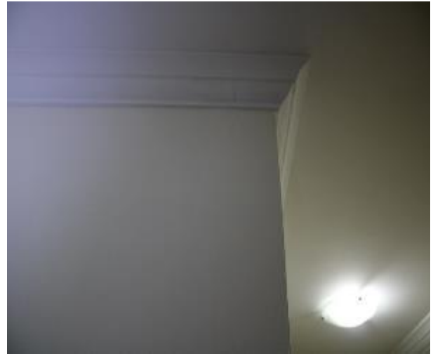
Figure 509 - Crack propagation through open kitchen/ lounge room internal wall
