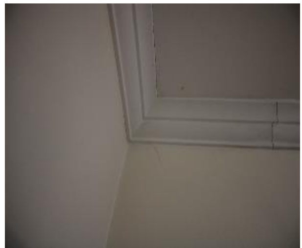
Figure 513 - Crack propagation through open kitchen/ lounge room ceiling
