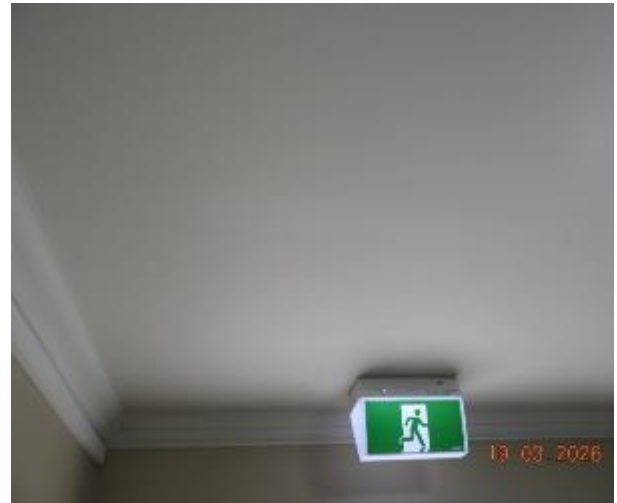
Figure 22 - General condition of level 1 common area ceiling
