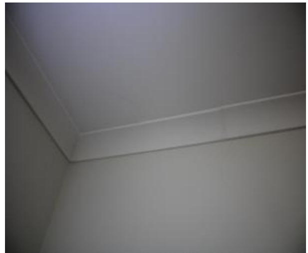
Figure 1002 - Crack propagation through study ceiling
