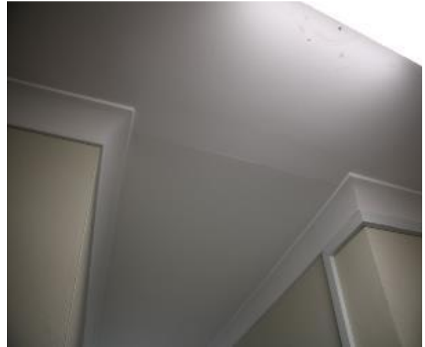
Figure 152 - General condition of level 5 common area ceiling
