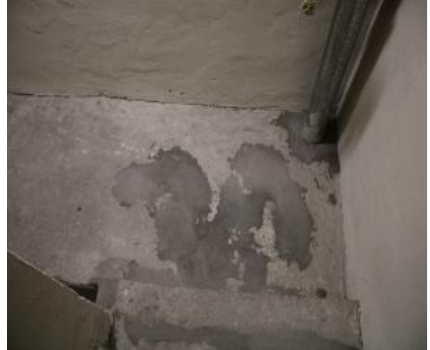
Figure 304 - General condition of level 5 to basement B2 fire stairs concrete floor
