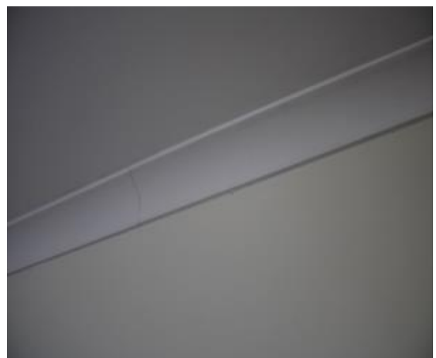
Figure 597 - Crack propagation through bedroom 2 ceiling
