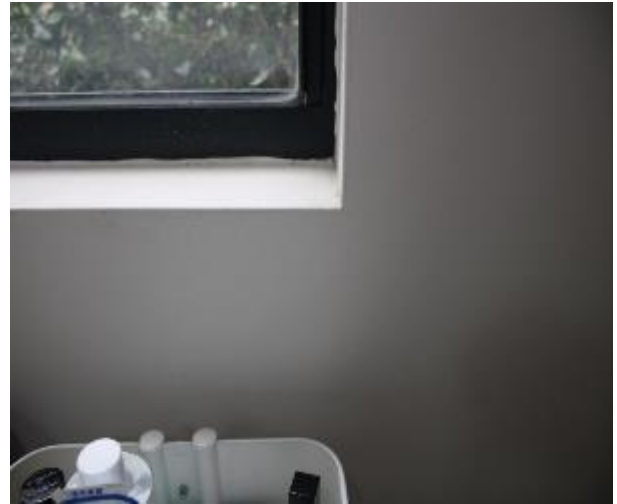
Figure 699 - Crack propagation through bedroom 1 internal wall
