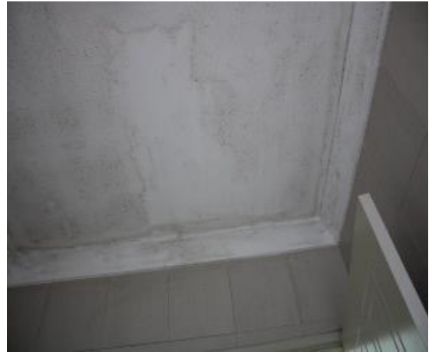
Figure 1357 - Water damage evident through bathroom 1 ceiling
