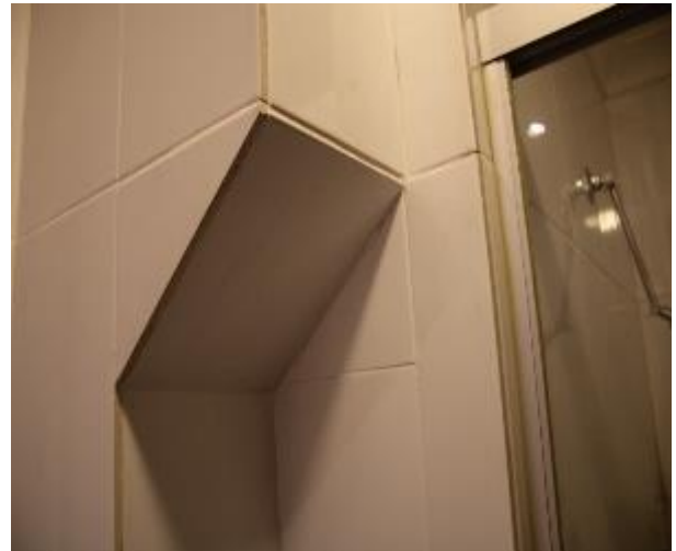
Figure 1149 - Crack propagation through ensuite bathroom internal wall
