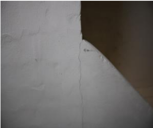
Figure 239 - Crack propagation through level 5 to basement B2 fire stairs internal wall
