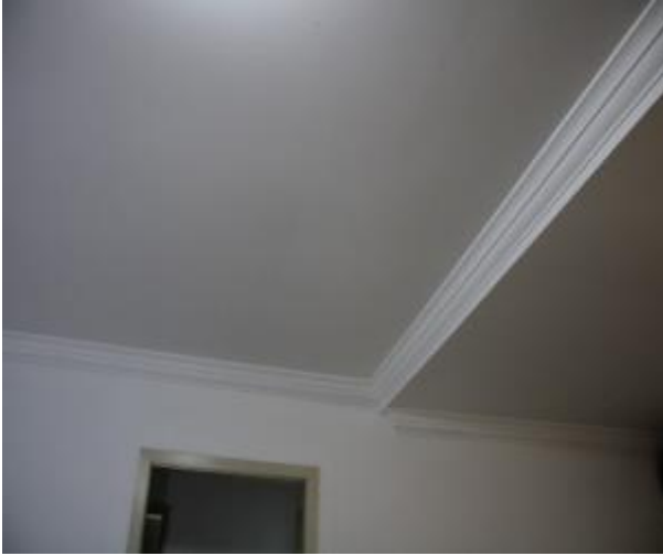
Figure 1278 - General condition of dining room ceiling
