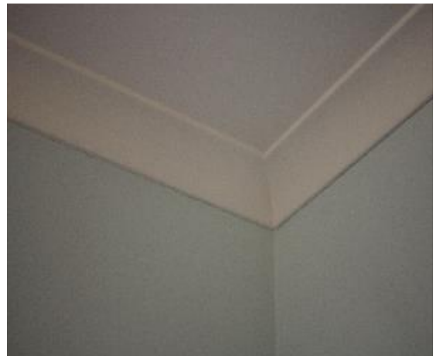
Figure 1181 - Crack propagation through bedroom 2 ceiling
