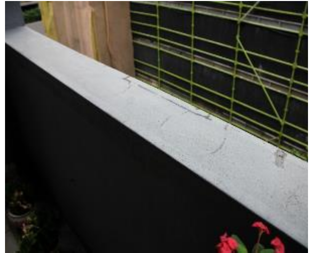
Figure 1072 - Crack propagation through external wall
