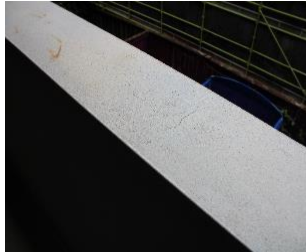
Figure 649 - Crack propagation through external wall
