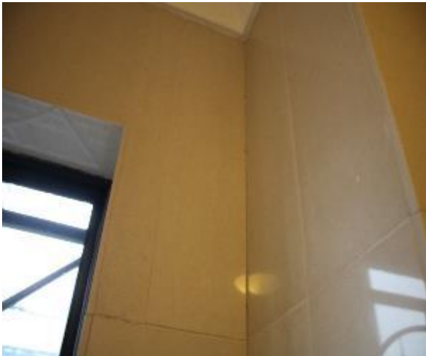
Figure 1037 - Crack propagation through bathroom 1 internal wall
