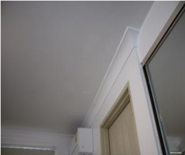
Figure 1370 - General condition of bedroom 2 ceiling
