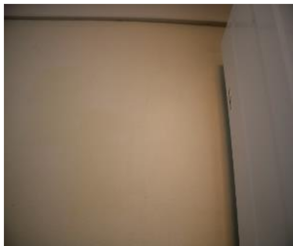
Figure 535 - Crack propagation through laundry internal wall
