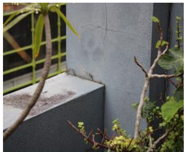
Figure 1585 - Crack propagation through external wall
