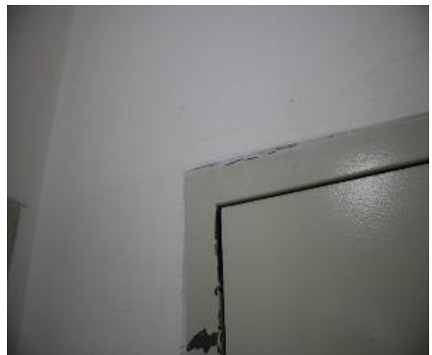
Figure 489 - Crack propagation through open kitchen/ lounge room internal wall
