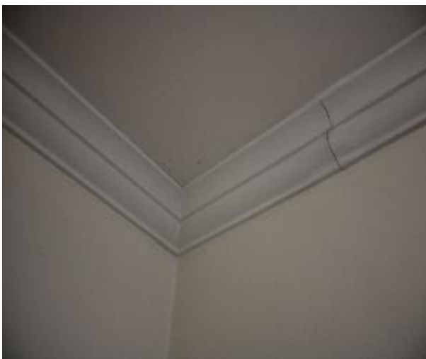
Figure 512 - Crack propagation through open kitchen/ lounge room ceiling
