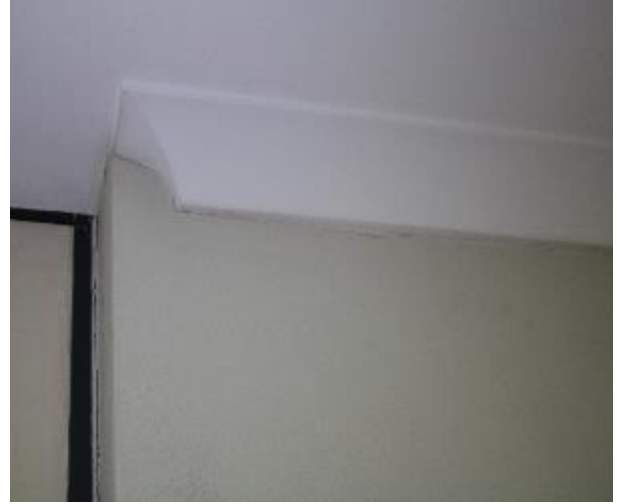
Figure 1563 - Crack propagation through bedroom 2 ceiling
