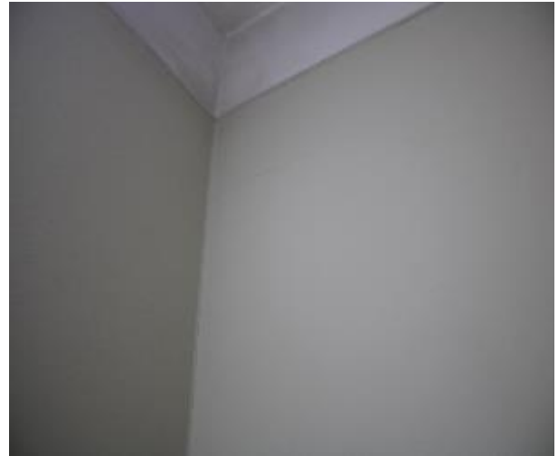
Figure 913 - Crack propagation through bedroom 3 internal wall
