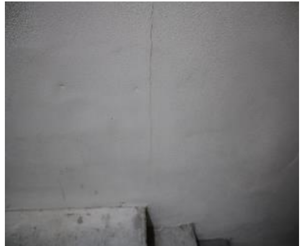
Figure 240 - Crack propagation through level 5 to basement B2 fire stairs internal wall
