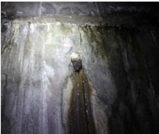
Figure 467 - Water damage evident through basement B2 fire stairs internal wall
