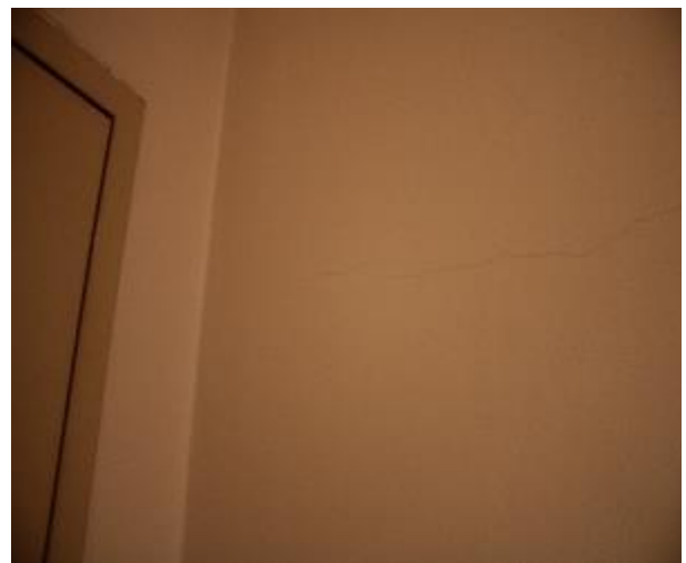
Figure 1091 - Crack propagation through lounge room internal wall
