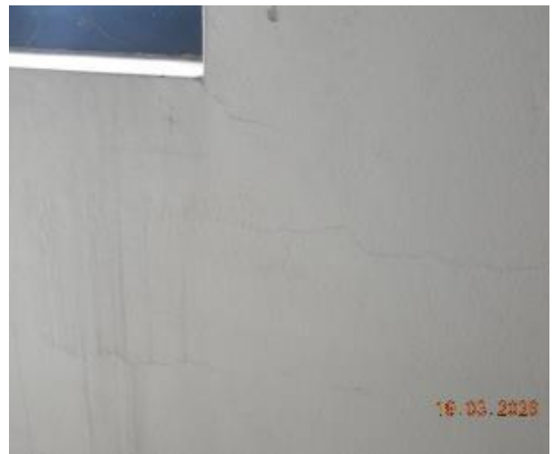
Figure 34 - Crack propagation through level 2 common area internal wall
