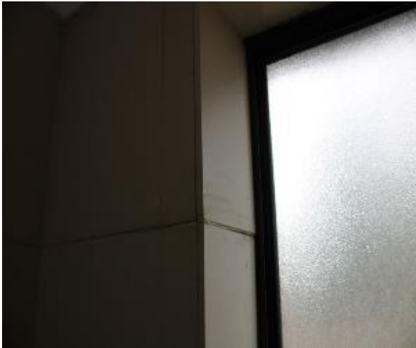
Figure 610 - Crack propagation through bathroom 1 internal wall
