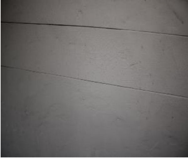
Figure 369 - Crack propagation through level 5 to basement B2 fire stairs internal wall
