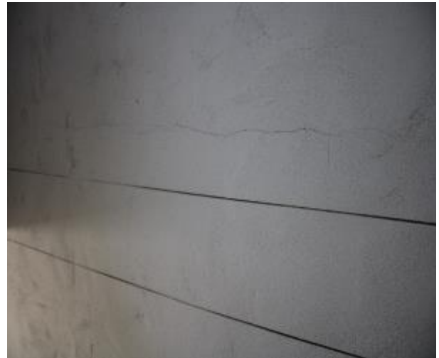
Figure 264 - Crack propagation through level 5 to basement B2 fire stairs internal wall
