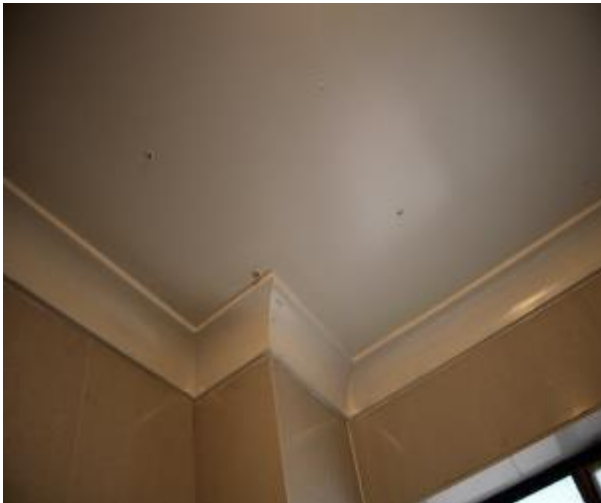
Figure 848 - General condition of bathroom 1 ceiling
