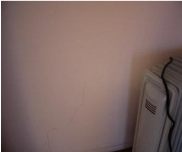
Figure 1128 - Crack propagation through bedroom 1 internal wall
