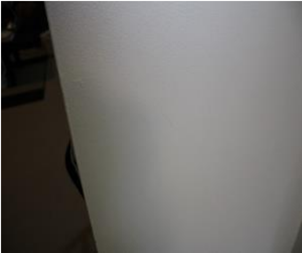
Figure 870 - Crack propagation through corridor internal wall
