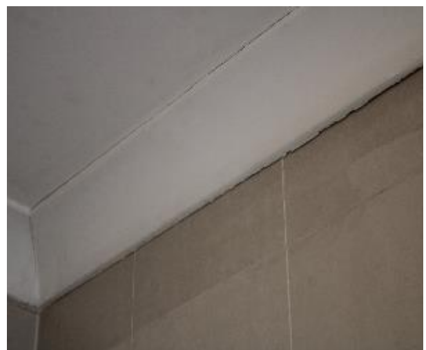
Figure 1543 - Crack propagation through bathroom 1 ceiling
