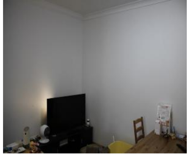
Figure 1273 - General condition of dining room internal wall
