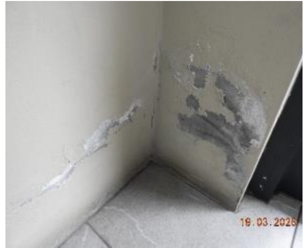
Figure 14 - Paint flaking through level 1 common area internal wall
