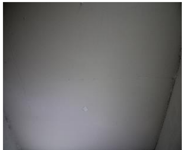
Figure 248 - Crack propagation through level 5 to basement B2 fire stairs underside slab
