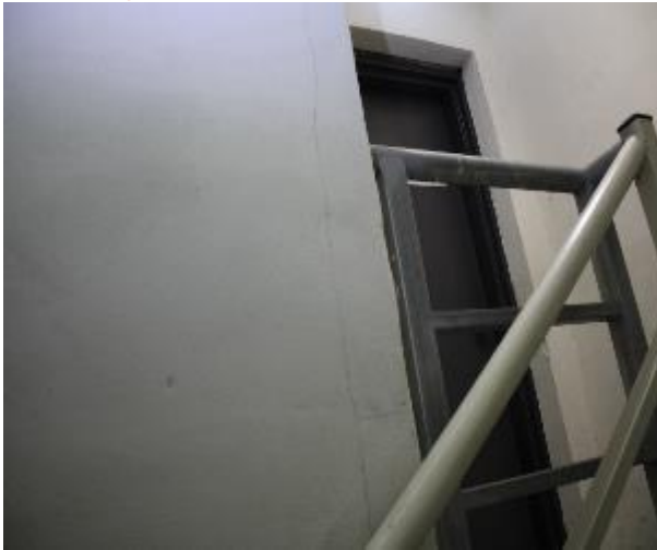
Figure 423 - Crack propagation through level 5 to basement B2 fire stairs internal wall
