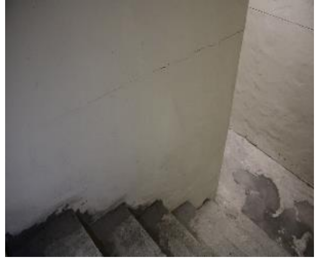
Figure 298 - Crack propagation through level 5 to basement B2 fire stairs internal wall
