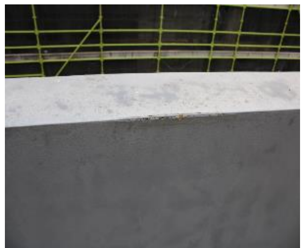
Figure 1307 - Crack propagation through external wall
