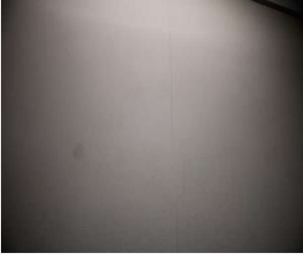
Figure 145 - Crack propagation through level 5 common area internal wall
