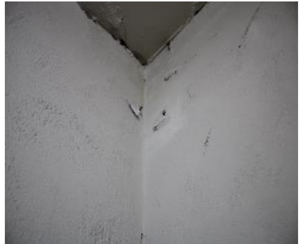
Figure 228 - Paint flaking through level 5 to basement B2 fire stairs internal wall
