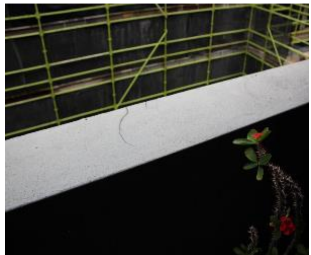
Figure 1070 - Crack propagation through external wall
