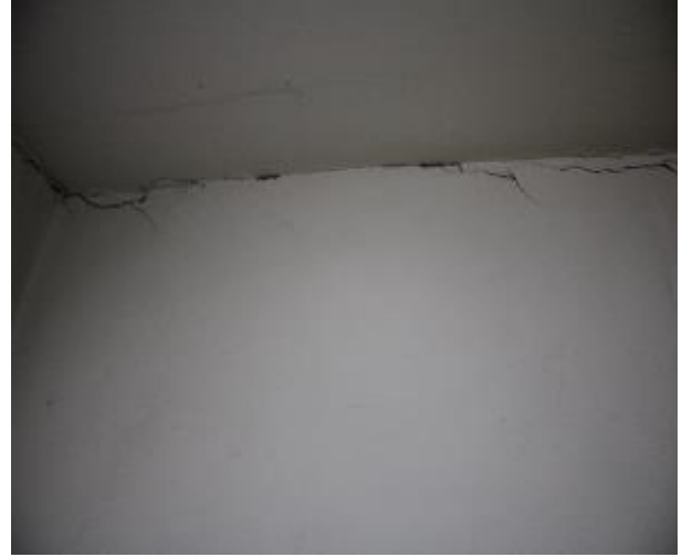
Figure 340 - Crack propagation through level 5 to basement B2 fire stairs internal wall
