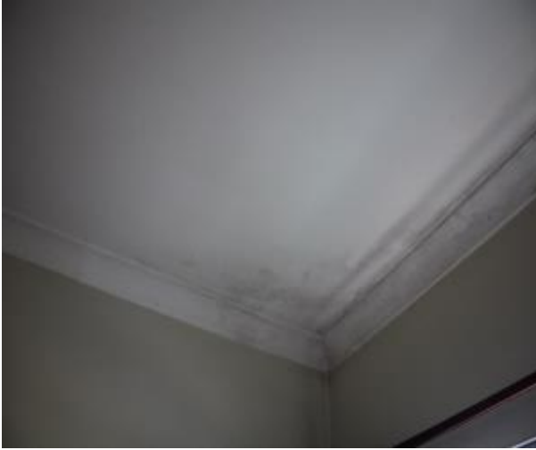
Figure 924 - Water damage evident through bedroom 3 ceiling
