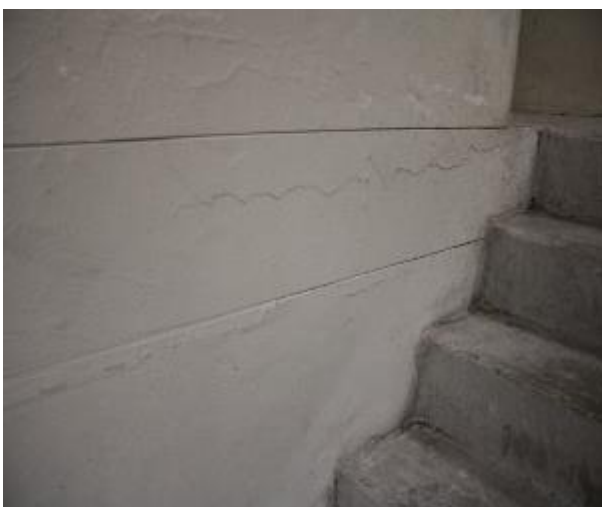
Figure 361 - Crack propagation through level 5 to basement B2 fire stairs internal wall
