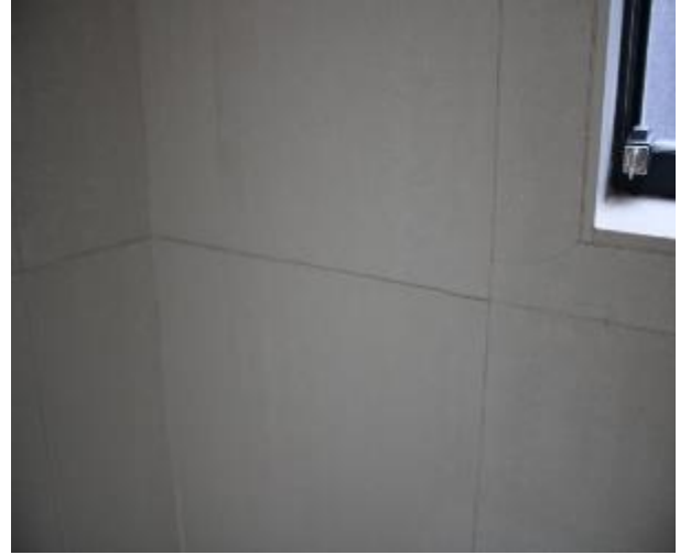
Figure 741 - Crack propagation through bathroom 1 internal wall
