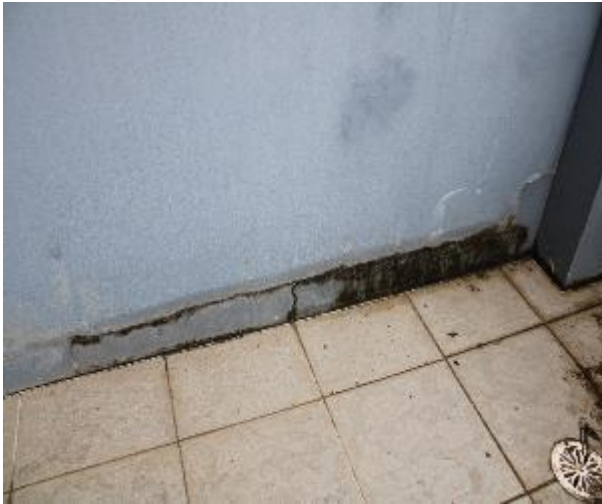
Figure 1314 - Crack propagation through external wall
