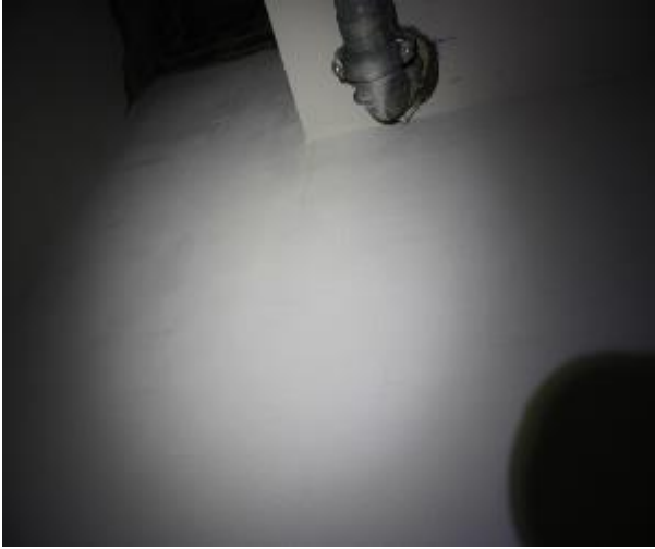
Figure 417 - Crack propagation through level 5 to basement B2 fire stairs internal wall
