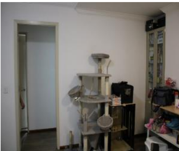
Figure 1270 - General condition of dining room internal wall
