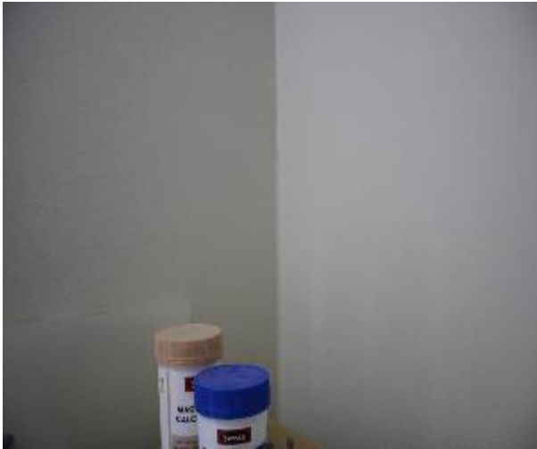
Figure 912 - Crack propagation through bedroom 3 internal wall
