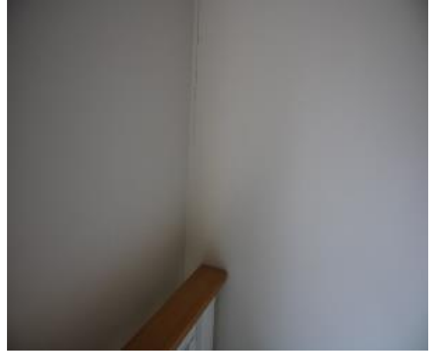
Figure 623 - Crack propagation through bedroom 3 internal wall
