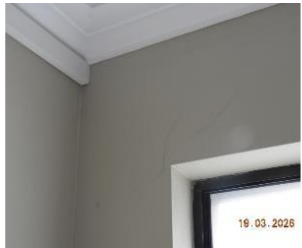
Figure 40 - Crack propagation through level 2 common area internal wall
