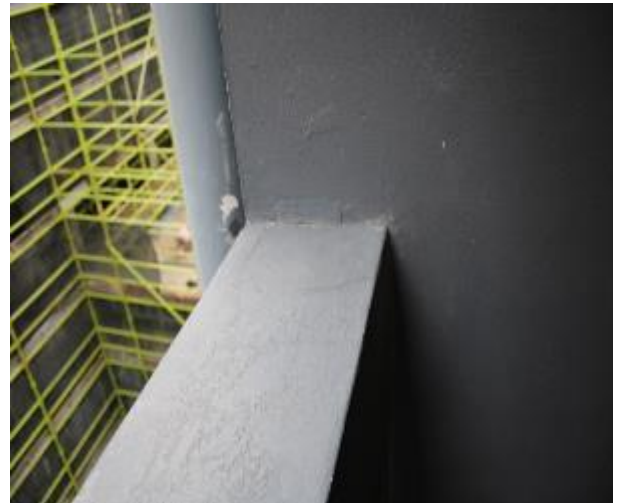
Figure 1221 - Crack propagation through external wall
