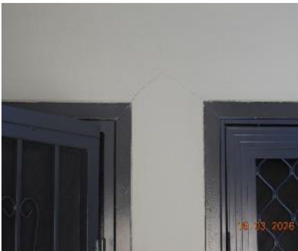
Figure 45 - Crack propagation through level 2 common area internal wall
