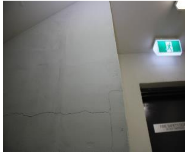
Figure 424 - Crack propagation through level 5 to basement B2 fire stairs internal wall
