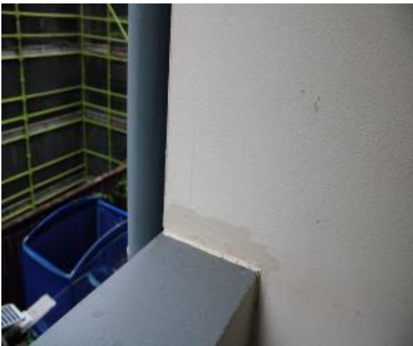
Figure 786 - Crack propagation through external wall
