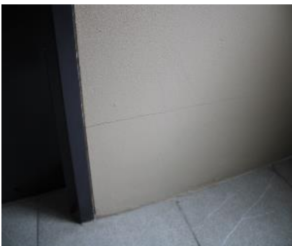
Figure 101 - Crack propagation through level 4 common area internal wall
