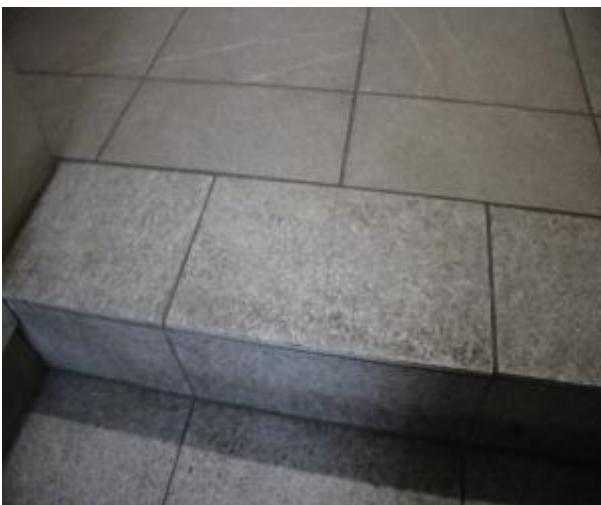
Figure 137 - Crack propagation through level 5 common area floor tiles
