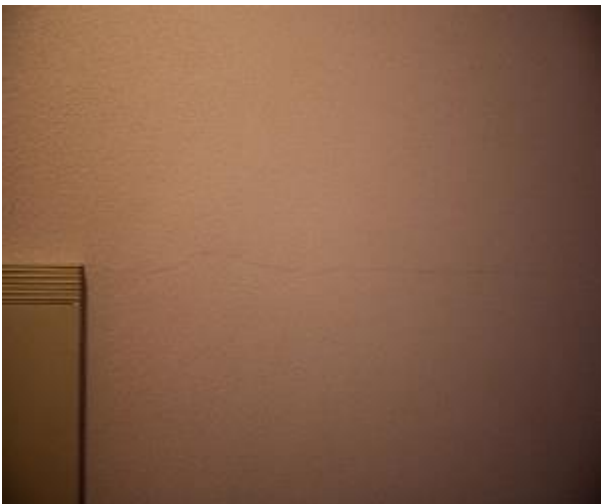
Figure 1120 - Crack propagation through bedroom 1 internal wall
