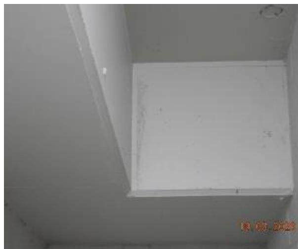
Figure 212 - General condition of B2 to Level 1 fire stairs underside slab
