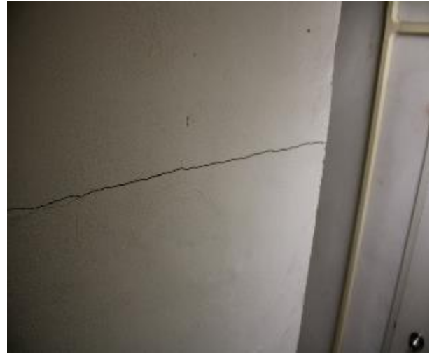
Figure 322 - Crack propagation through level 5 to basement B2 fire stairs internal wall
