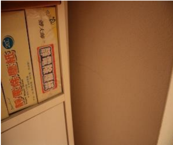
Figure 1086 - Crack propagation through lounge room internal wall
