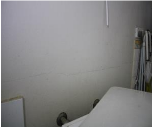
Figure 1436 - Crack propagation through laundry internal wall
