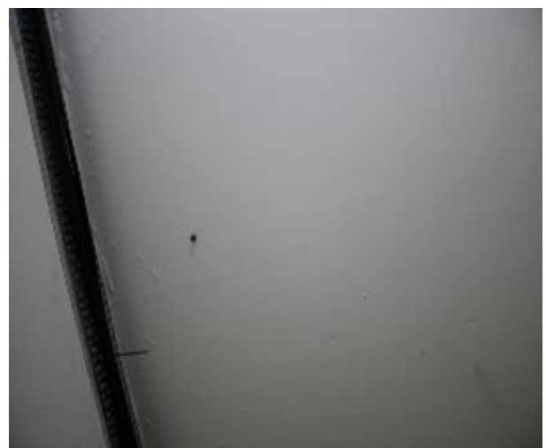
Figure 428 - Crack propagation through level 5 to basement B2 fire stairs underside stairs
