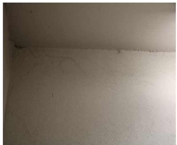
Figure 314 - Crack propagation through level 5 to basement B2 fire stairs internal wall
