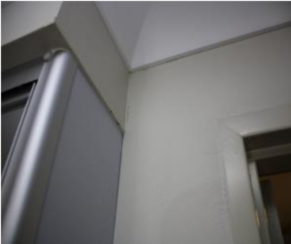
Figure 1478 - Crack propagation through bedroom 1 internal wall
