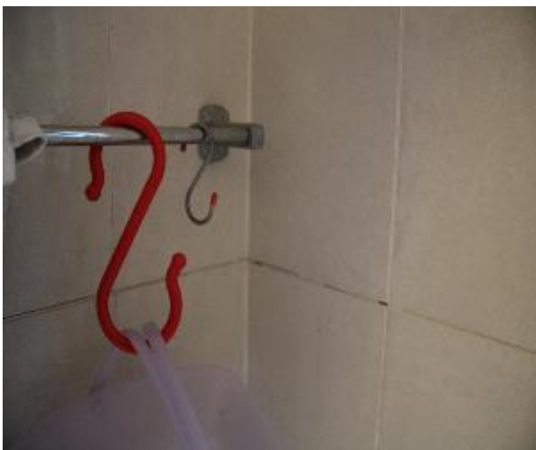
Figure 1039 - Crack propagation through bathroom 1 internal wall
