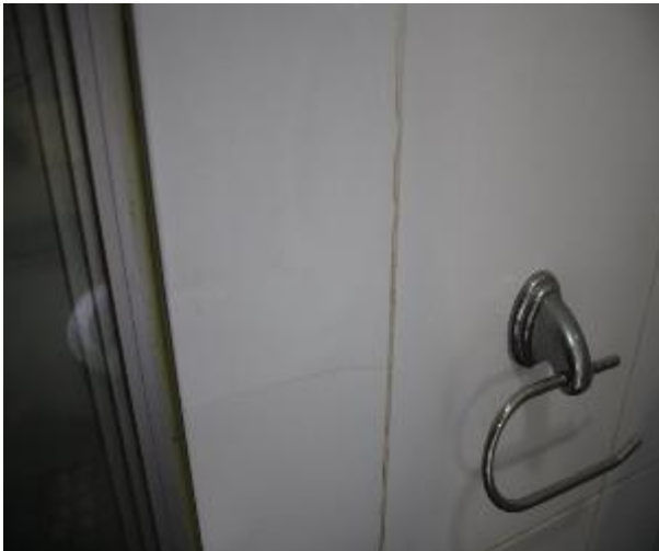
Figure 564 - Crack propagation through ensuite bathroom internal wall
