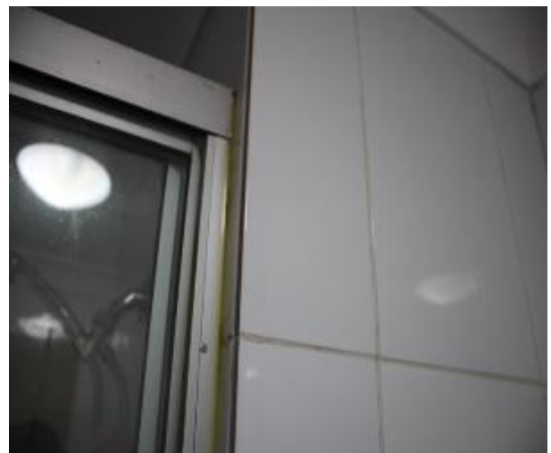
Figure 567 - Crack propagation through ensuite bathroom internal wall
