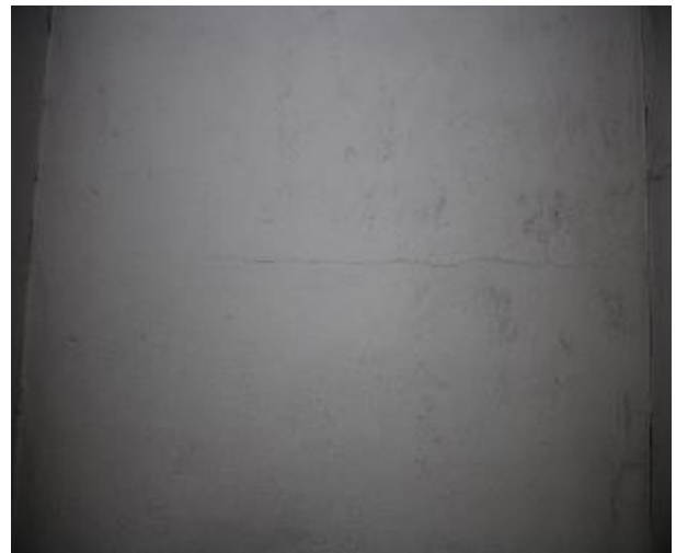
Figure 290 - Crack propagation through level 5 to basement B2 fire stairs internal wall
