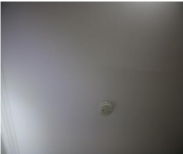
Figure 1276 - General condition of dining room ceiling
