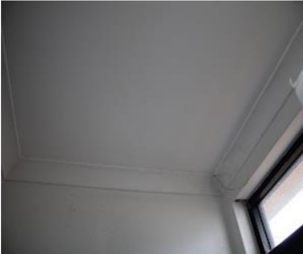
Figure 1268 - General condition of laundry ceiling
