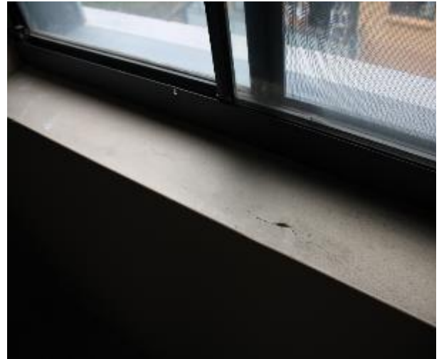
Figure 98 - Crack propagation through level 4 common area internal wall
