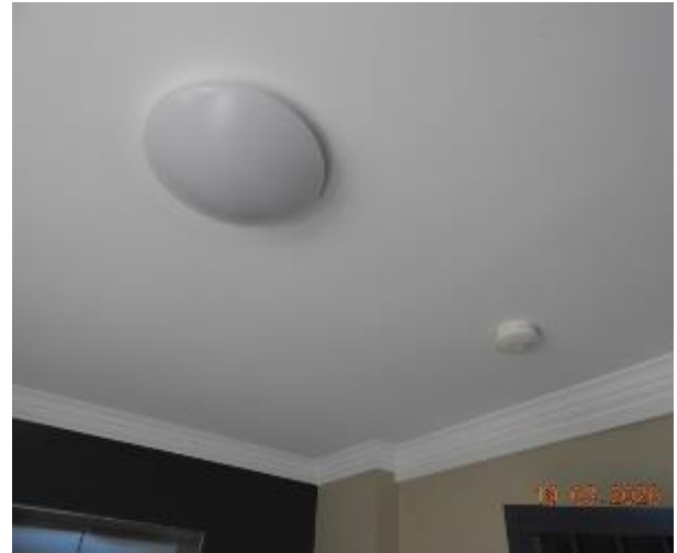
Figure 50 - General condition of level 2 common area ceiling
