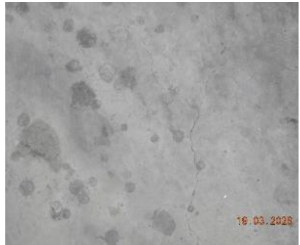
Figure 192 - Crack propagation through B2 to Level 1 fire stairs pavement slab
