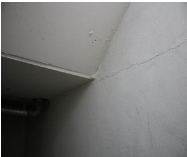
Figure 425 - Crack propagation through level 5 to basement B2 fire stairs internal wall
