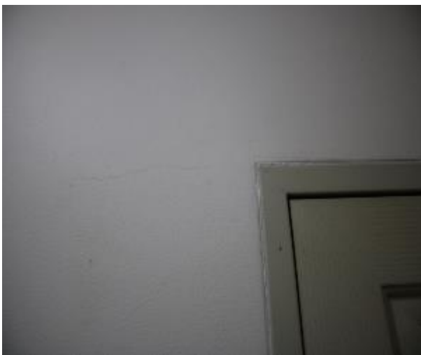
Figure 488 - Crack propagation through open kitchen/ lounge room internal wall
