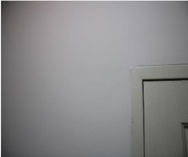
Figure 810 - Crack propagation through open kitchen/ lounge room internal wall
