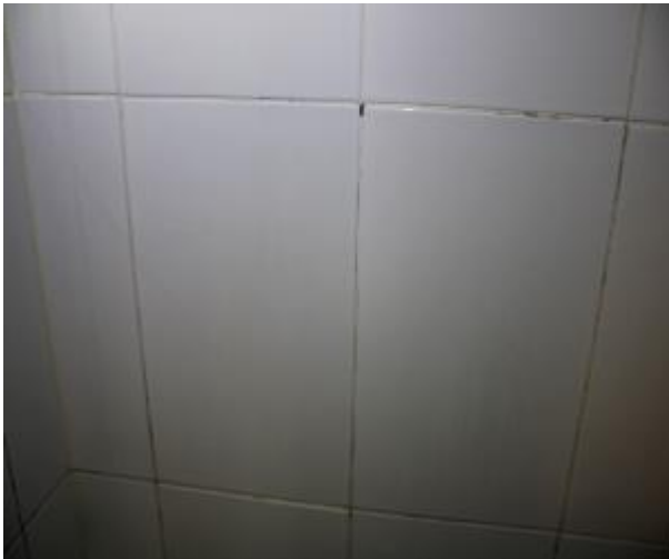
Figure 718 - Crack propagation through ensuite bathroom internal wall
