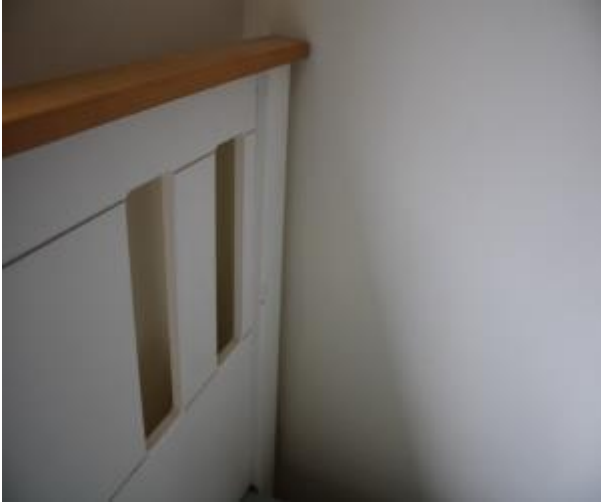
Figure 622 - Crack propagation through bedroom 3 internal wall
