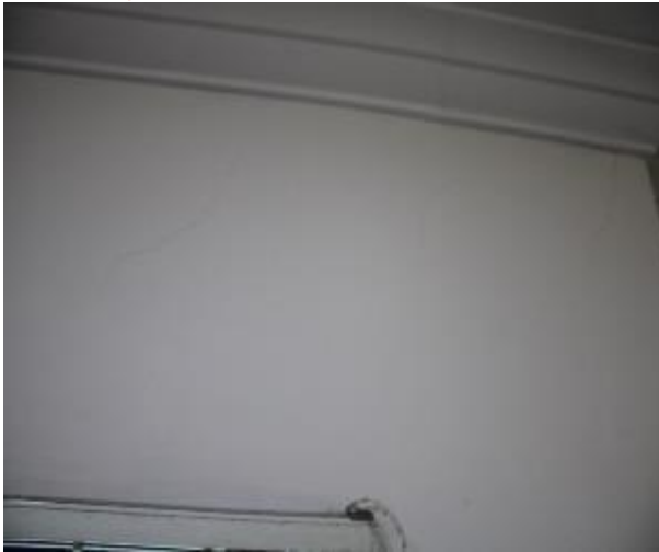
Figure 496 - Crack propagation through open kitchen/ lounge room internal wall
