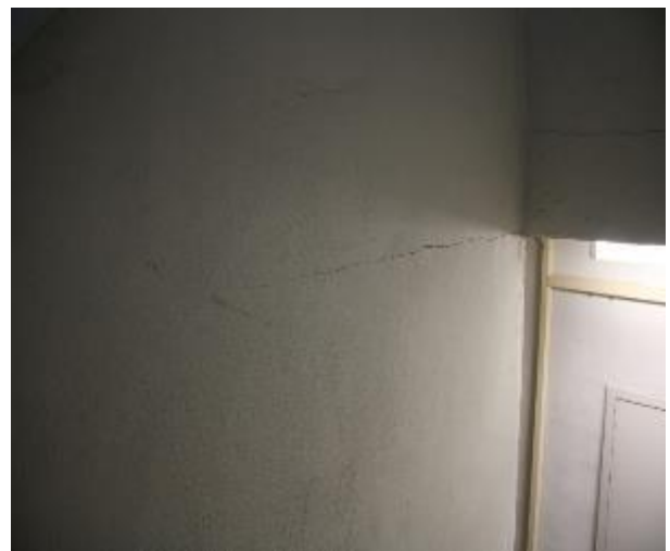
Figure 272 - Crack propagation through level 5 to basement B2 fire stairs internal wall
