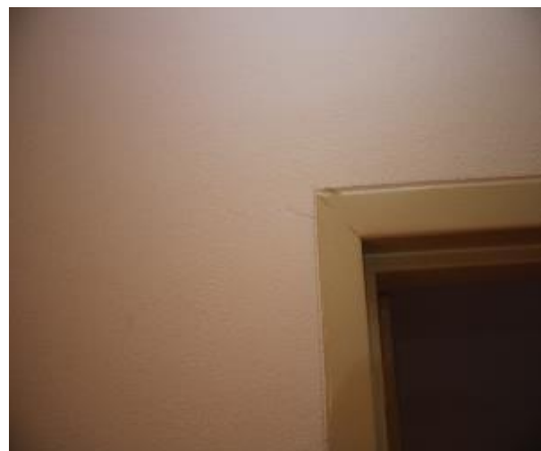
Figure 1095 - Crack propagation through lounge room internal wall
