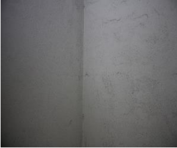
Figure 267 - Crack propagation through level 5 to basement B2 fire stairs internal wall
