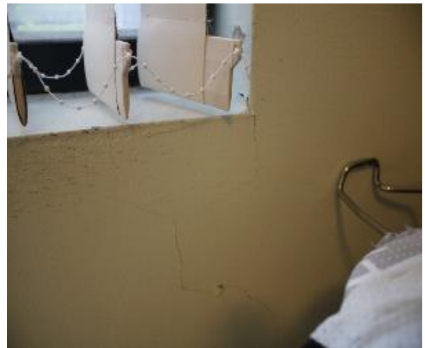
Figure 1167 - Crack propagation through bedroom 2 internal wall
