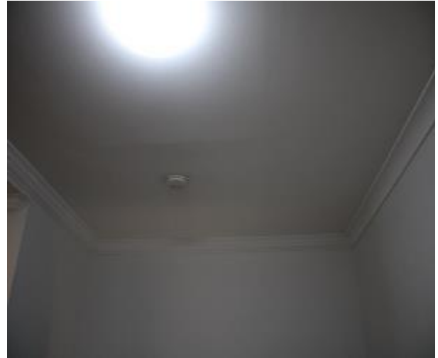
Figure 1275 - General condition of dining room ceiling
