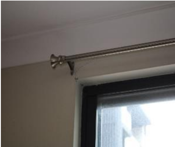
Figure 1472 - Crack propagation through bedroom 1 internal wall
