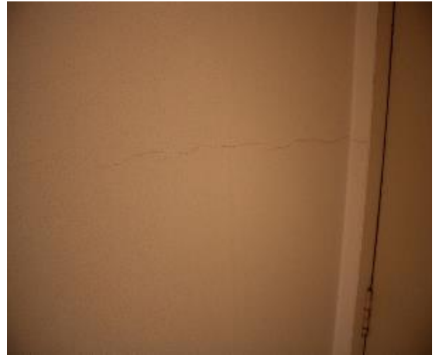
Figure 1087 - Crack propagation through lounge room internal wall
