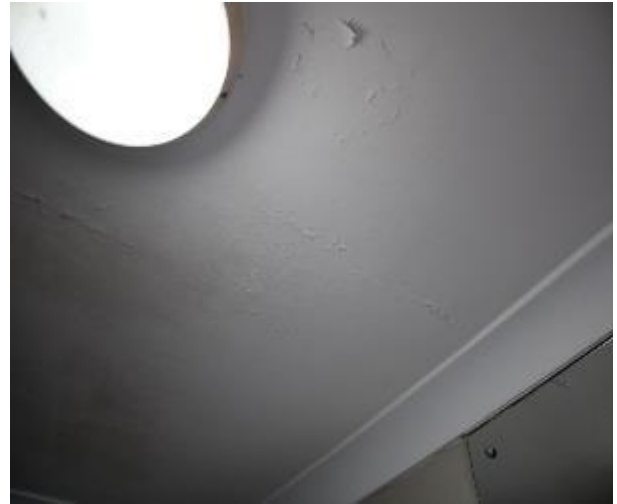
Figure 617 - Paint flaking through bathroom 1 ceiling
