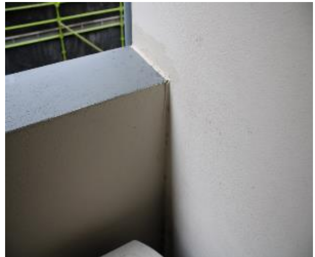
Figure 785 - Crack propagation through external wall
