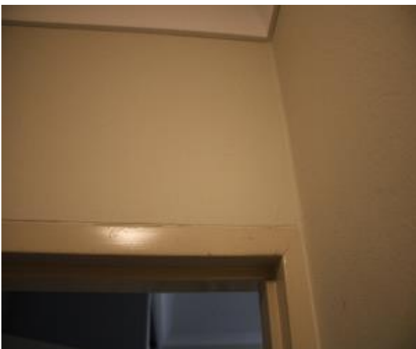
Figure 898 - Crack propagation through corridor internal wall
