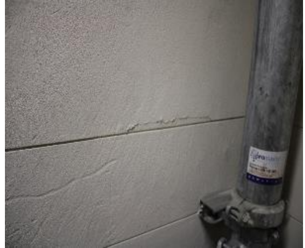
Figure 364 - Crack propagation through level 5 to basement B2 fire stairs internal wall
