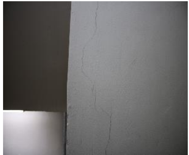
Figure 342 - Crack propagation through level 5 to basement B2 fire stairs internal wall
