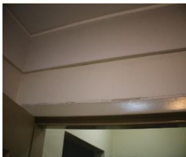
Figure 537 - Crack propagation through laundry internal wall
