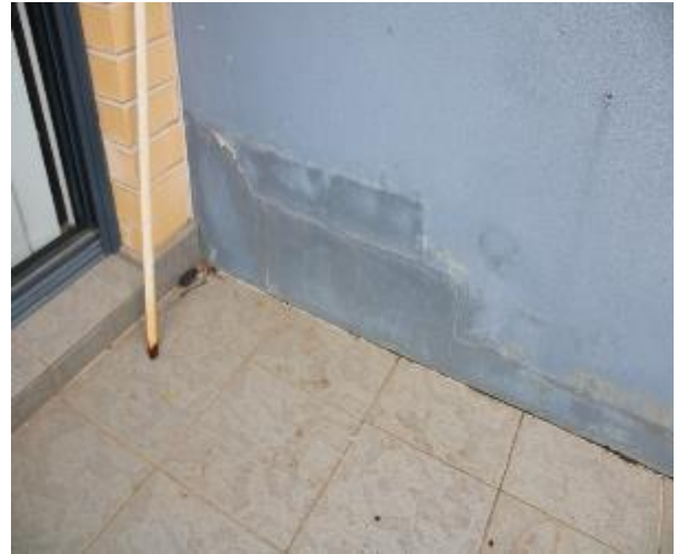
Figure 1315 - Crack propagation through external wall
