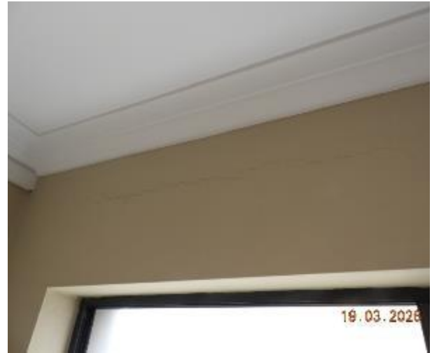
Figure 62 - Crack propagation through level 3 common area internal wall
