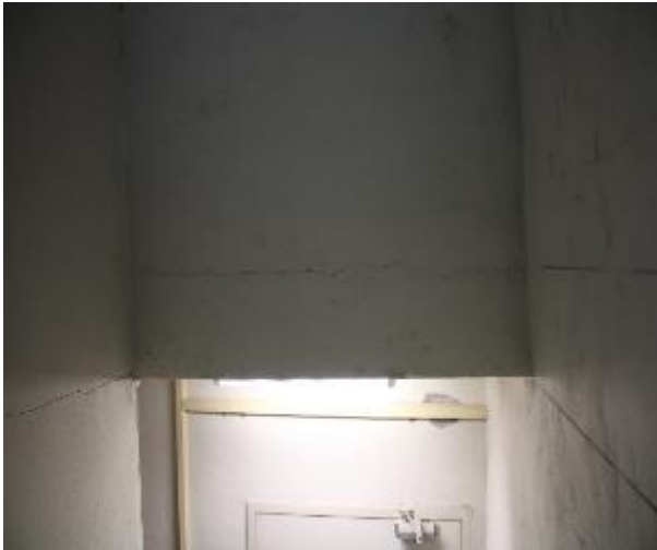
Figure 273 - Crack propagation through level 5 to basement B2 fire stairs internal wall
