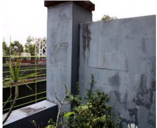
Figure 1581 - Crack propagation through external wall
