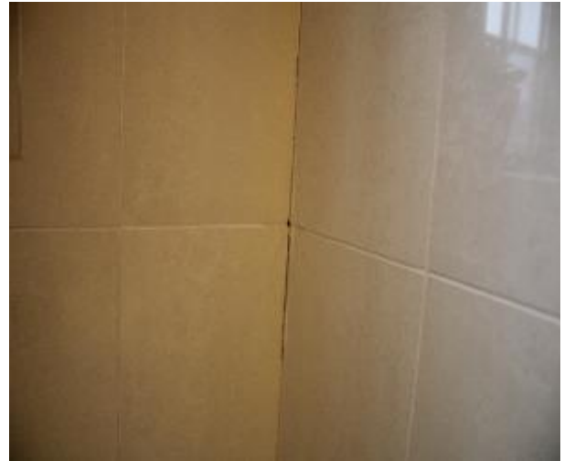
Figure 1036 - Crack propagation through bathroom 1 internal wall
