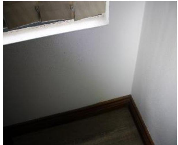
Figure 1329 - Crack propagation through study internal wall
