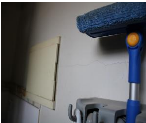
Figure 1440 - Crack propagation through laundry internal wall
