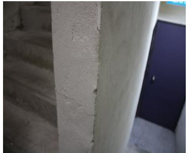
Figure 378 - Crack propagation through level 5 to basement B2 fire stairs internal wall
