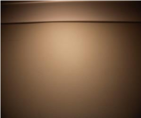
Figure 894 - Crack propagation through corridor internal wall
