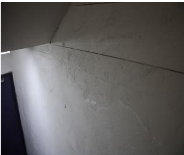
Figure 373 - Crack propagation through level 5 to basement B2 fire stairs internal wall
