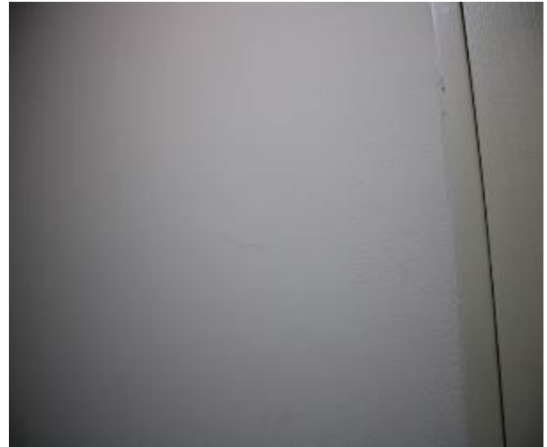
Figure 811 - Crack propagation through open kitchen/ lounge room internal wall
