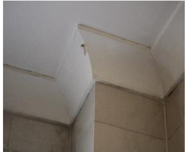
Figure 1545 - Crack propagation and paint flaking through bathroom 1 ceiling
