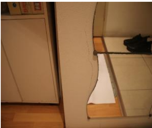
Figure 1084 - Crack propagation through lounge room internal wall
