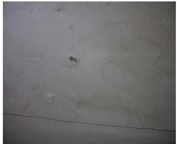
Figure 258 - Crack propagation through level 5 to basement B2 fire stairs internal wall
