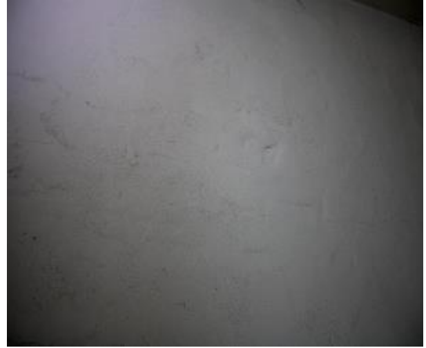
Figure 268 - Crack propagation through level 5 to basement B2 fire stairs internal wall
