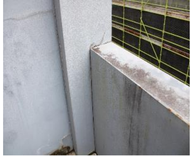
Figure 1309 - Crack propagation through external wall
