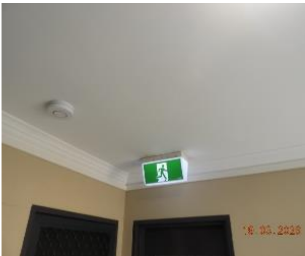
Figure 81 - General condition of level 3 common area ceiling
