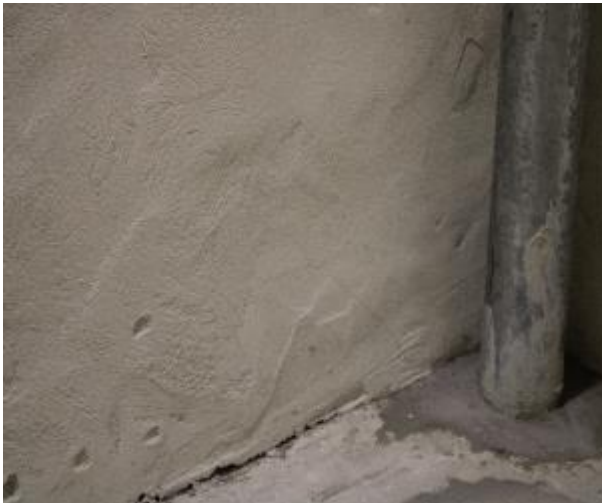
Figure 311 - Crack propagation through level 5 to basement B2 fire stairs internal wall
