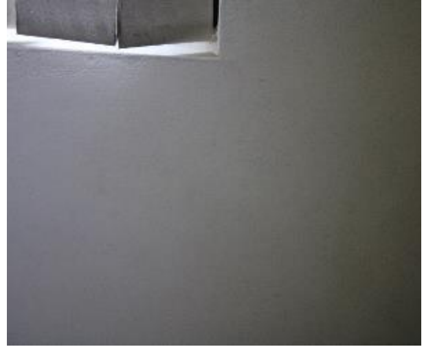
Figure 587 - Crack propagation through bedroom 2 internal wall
