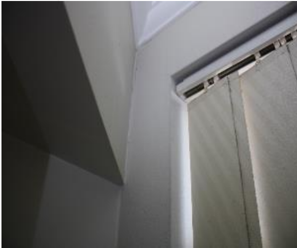
Figure 1424 - Crack propagation through kitchen internal wall
