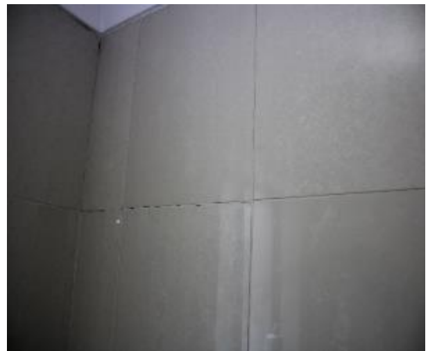
Figure 607 - Crack propagation through bathroom 1 internal wall
