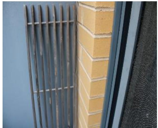
Figure 1579 - Crack propagation through external wall
