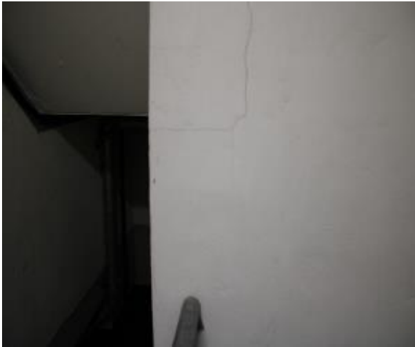
Figure 399 - Crack propagation through level 5 to basement B2 fire stairs internal wall
