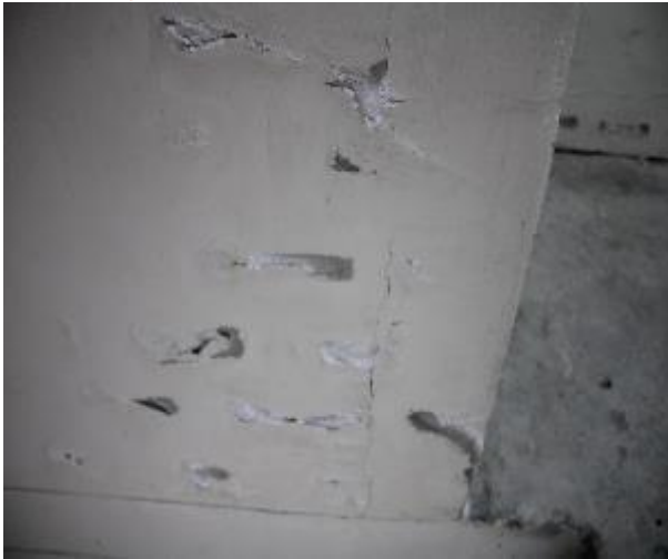
Figure 255 - Crack propagation and paint flaking through level 5 to basement B2 fire stairs internal wall
