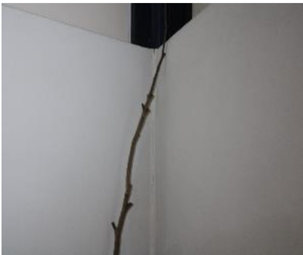
Figure 1552 - Crack propagation through bedroom 2 internal wall
