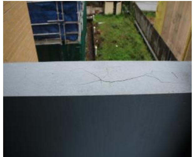
Figure 1074 - Crack propagation through external wall
