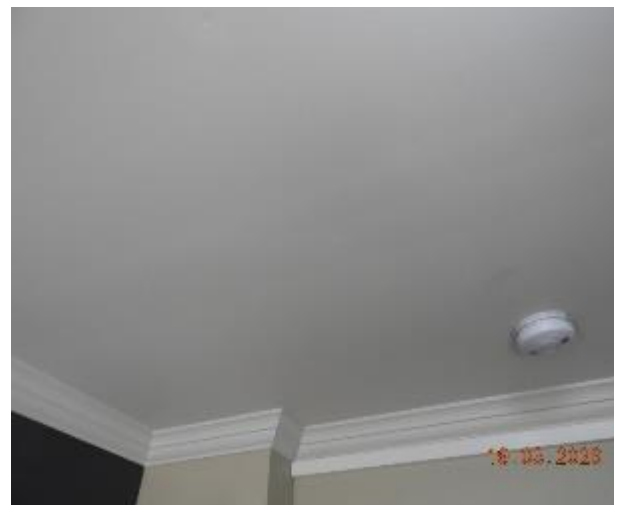
Figure 24 - General condition of level 1 common area ceiling
