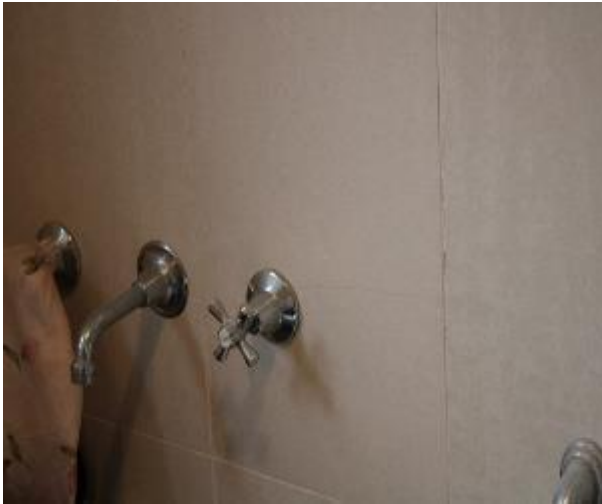
Figure 840 - Crack propagation through bathroom 1 internal wall
