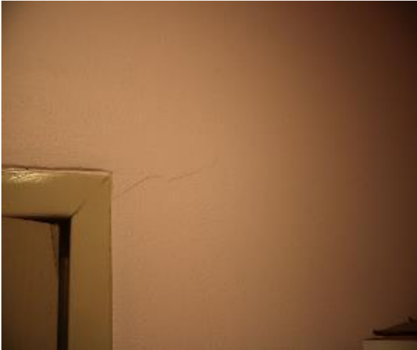
Figure 1124 - Crack propagation through bedroom 1 internal wall
