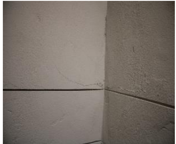
Figure 318 - Crack propagation through level 5 to basement B2 fire stairs internal wall
