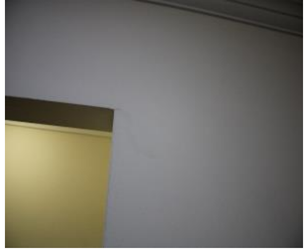
Figure 503 - Crack propagation through open kitchen/ lounge room internal wall
