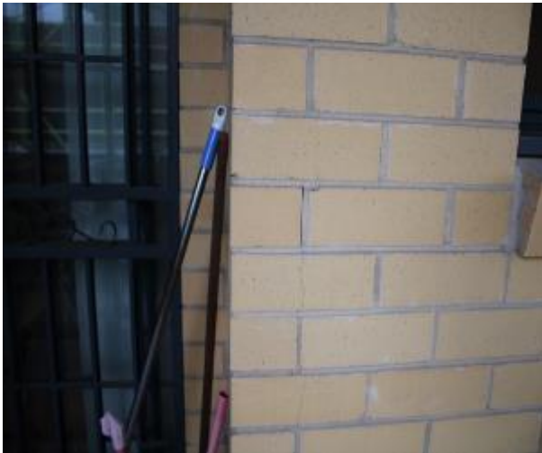
Figure 1232 - Crack propagation through external wall
