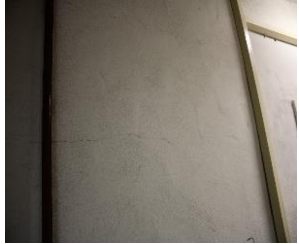
Figure 286 - Crack propagation through level 5 to basement B2 fire stairs internal wall
