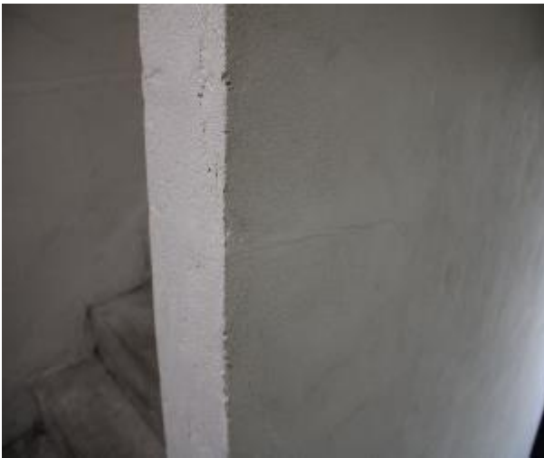
Figure 377 - Crack propagation through level 5 to basement B2 fire stairs internal wall
