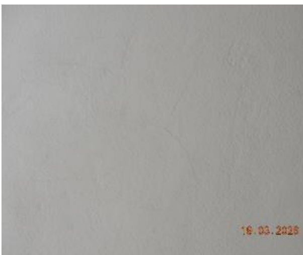
Figure 35 - Crack propagation through level 2 common area internal wall
