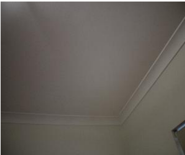
Figure 1027 - General condition of bedroom 1 ceiling
