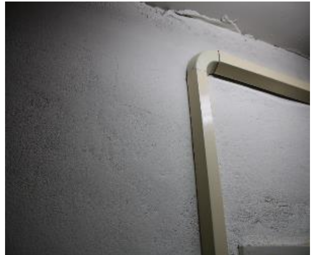
Figure 234 - Crack propagation through level 5 to basement B2 fire stairs internal wall
