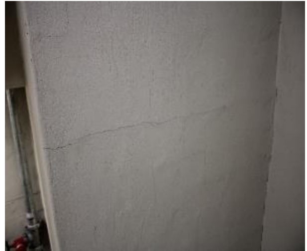
Figure 292 - Crack propagation through level 5 to basement B2 fire stairs internal wall
