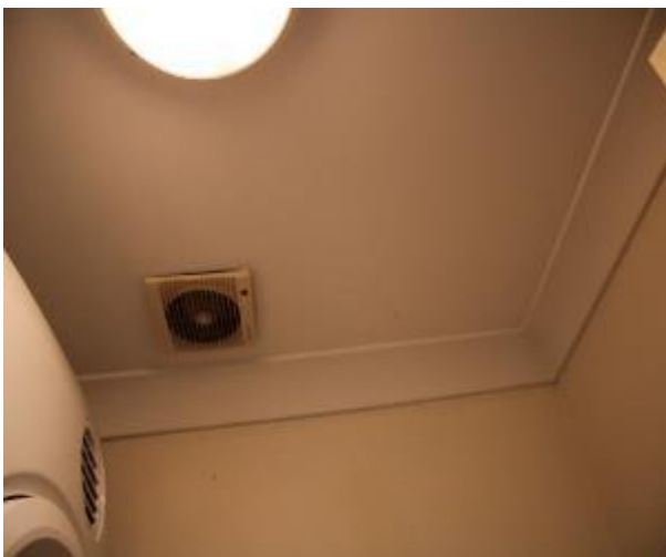
Figure 542 - General condition of laundry ceiling
