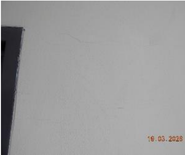
Figure 19 - Crack propagation through level 1 common area internal wall
