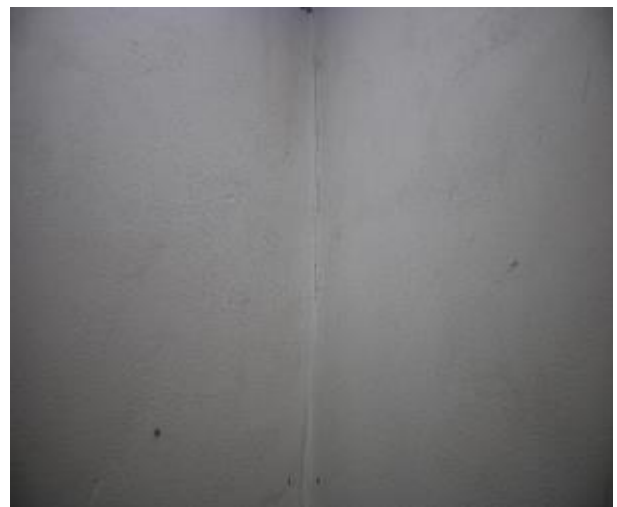
Figure 338 - Crack propagation through level 5 to basement B2 fire stairs internal wall
