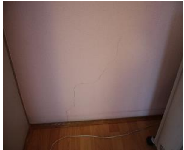
Figure 1127 - Crack propagation through bedroom 1 internal wall
