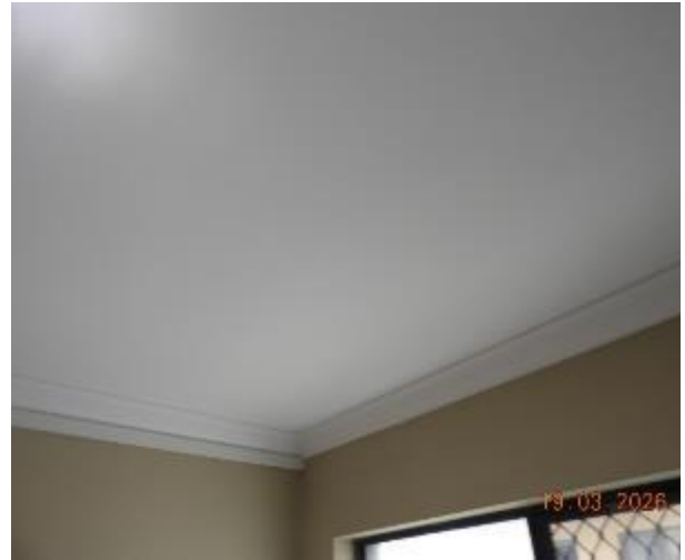
Figure 80 - General condition of level 3 common area ceiling
