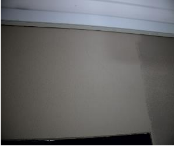
Figure 103 - Crack propagation through level 4 common area internal wall
