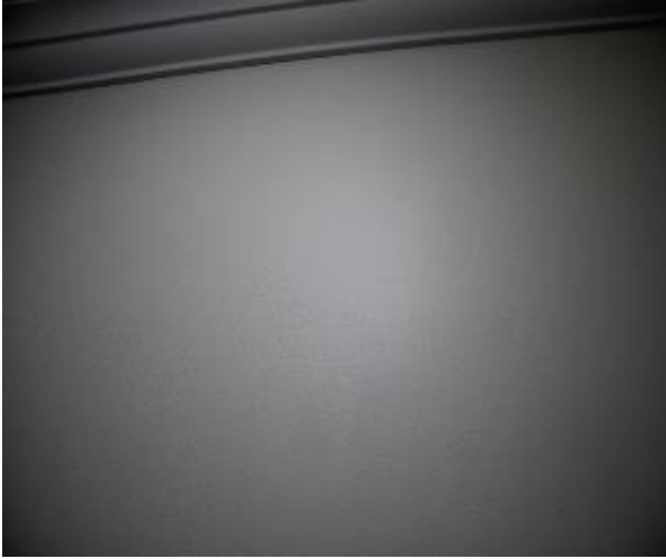
Figure 490 - Crack propagation through open kitchen/ lounge room internal wall
