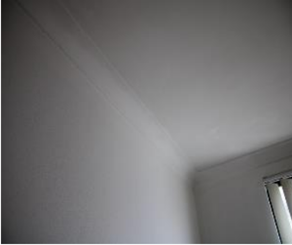
Figure 1368 - General condition of bedroom 2 ceiling
