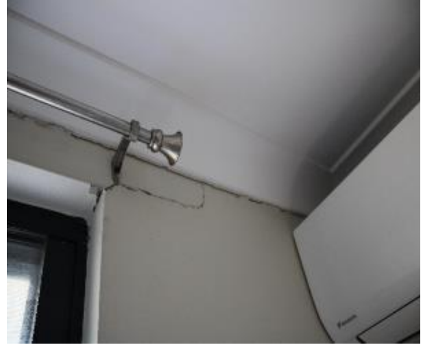
Figure 1491 - Crack propagation through bedroom 1 ceiling
