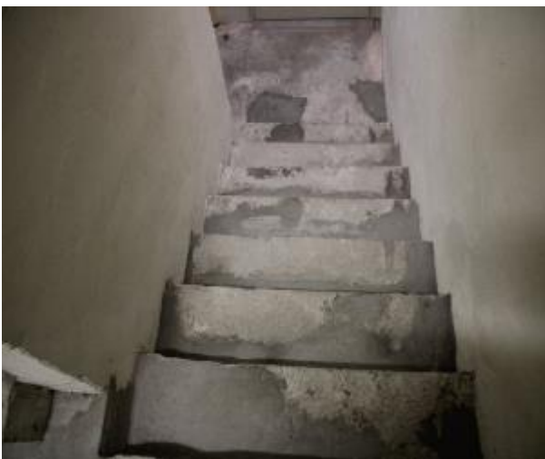
Figure 307 - General condition of level 5 to basement B2 fire stairs concrete floor
