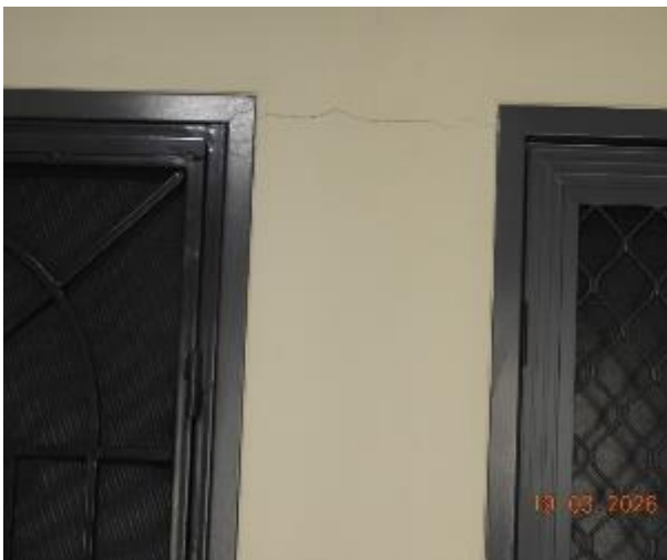
Figure 75 - Crack propagation through level 3 common area internal wall
