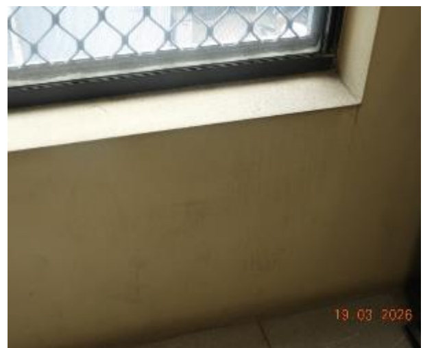
Figure 66 - Crack propagation through level 3 common area internal wall
