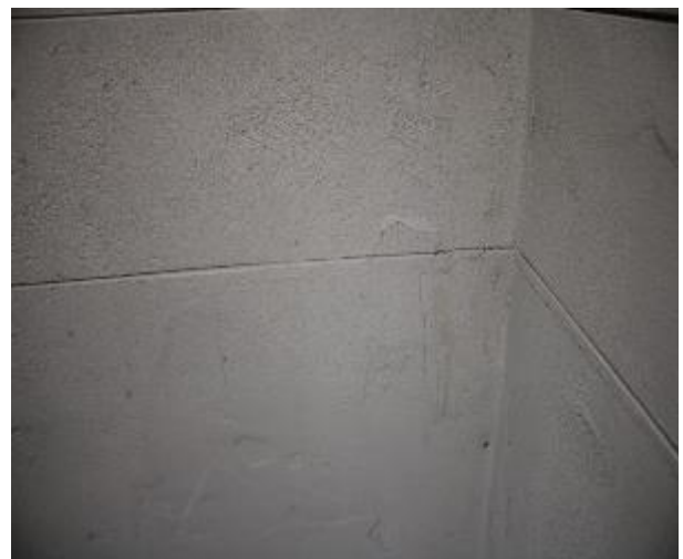
Figure 368 - Crack propagation through level 5 to basement B2 fire stairs internal wall
