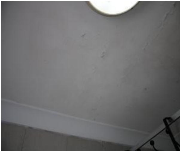
Figure 618 - Paint flaking through bathroom 1 ceiling
