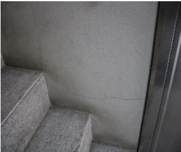
Figure 105 - Crack propagation through level 4 common area internal wall
