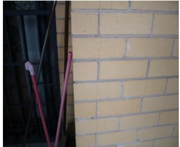
Figure 1231 - Crack propagation through external wall
