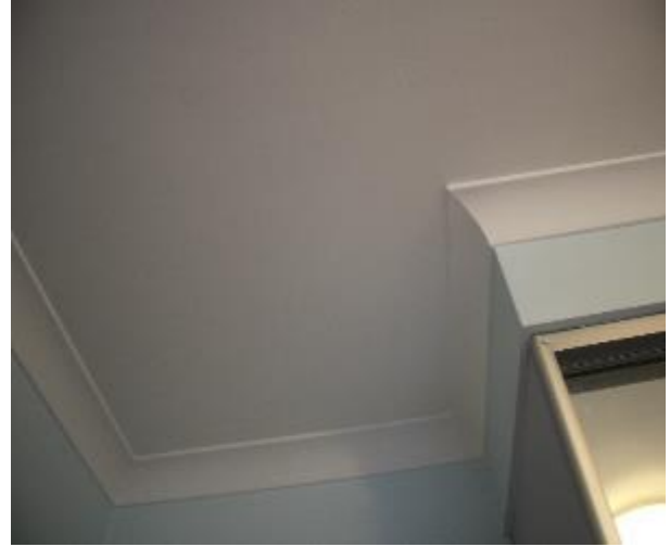
Figure 1177 - General condition of bedroom 2 ceiling
