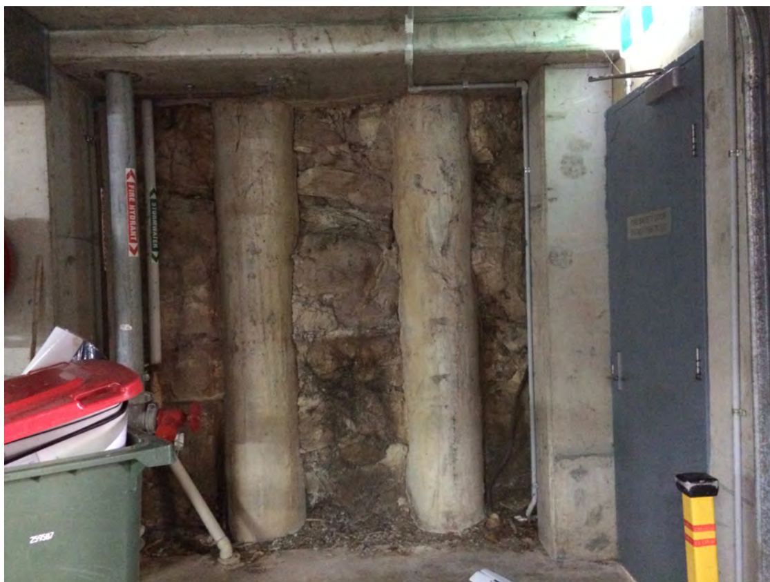
Photo 1: Northern wall east end – 1 of 5
