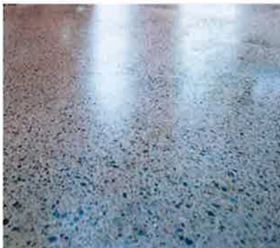
CFP-CONCRETE FLOOR POLISHED FINISH.
