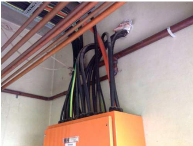
Photo No: J128740-003-HEAL-Photo011 Result: SMF - Presumed Positive Building/Level: Health Services Building-Level One Room/Location: Plant Room-Southeast Feature/Material: Penetrations-Pillow Insulation
