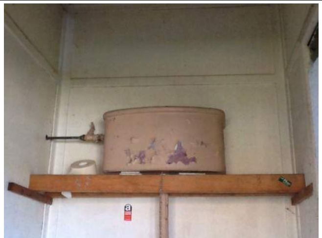
Photo No: J128740-002-ABOR-Photo017 Result: Asbestos - Positive Building/Level: Main Building-Basement Room/Location: Toilets- Feature/Material: Toilet Cistern-Packing
