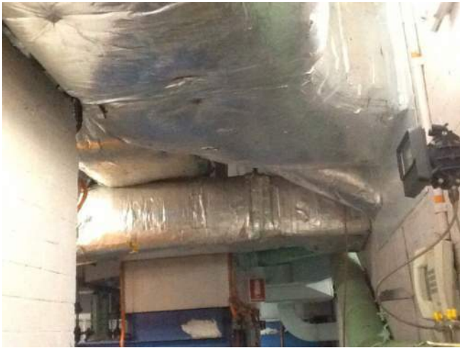
Photo No: J128740-001-MAND-Photo002 Result: SMF - Positive Building/Level: Main Building-All Levels Room/Location: All areas-Throughout Feature/Material: Ductwork Insulation-Insulation Material
