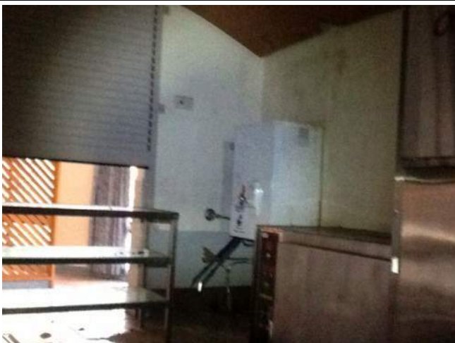
Photo No: J128740-001-MAND-Photo037 Result: SMF - Presumed Positive Building/Level: Main Building-Level One Room/Location: Dining Kitchen-Northeast Feature/Material: Boiler Insulation-Insulation Material
