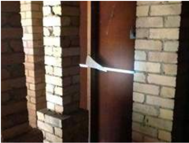
Photo No: J128740-002-ABOR-Photo102 Result: Asbestos - Presumed Positive Building/Level: Main Building-Sub-Floor Room/Location: North of Toilets-Behind Masonite Walls (accessible through Northern side) Feature/Material: Wall Cladding-Fibre Cement Sheetting
