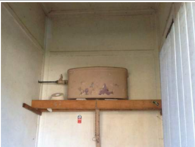
Photo No: J128740-002-ABOR-Photo020 Result: Lead (Paint) - Positive Building/Level: Main Building-Basement Room/Location: Toilet- Feature/Material: Plant & Equipment-Paint System/s
