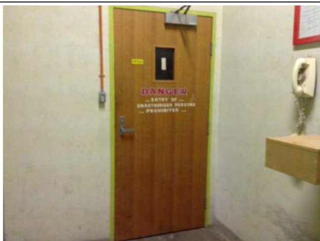
Photo No: J128740-003-HEAL-Photo007 Result: Asbestos - Positive Building/Level: Health Services Building-Level One Room/Location: Lift Motor Room-At Entrance Feature/Material: Fire Door-Fire Door Core
