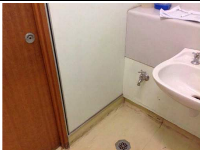
Photo No: J128740-003-HEAL-Photo021 Result: Asbestos - Positive Building/Level: Health Services Building-Level Three Room/Location: Finance Toilet-North and East Feature/Material: Wall-Fibre Cement Sheetting
