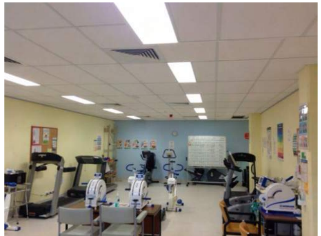
Photo No: J128740-003-HEAL-Photo031 Result: SMF - Presumed Positive Building/Level: Health Services Building-Level Two Room/Location: Physio and OT Treatment Area-Throughout Feature/Material: Ceiling Tiles-Insulation Material
