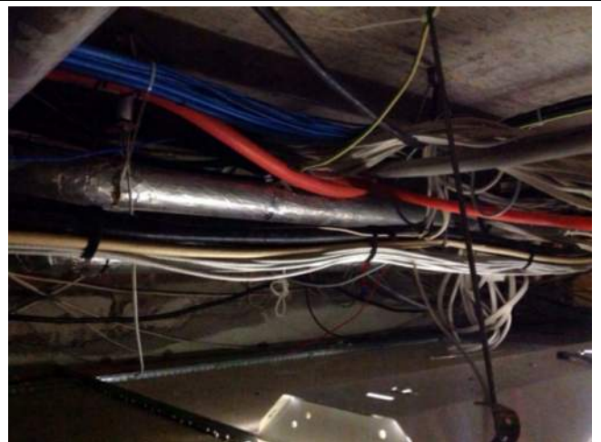
Photo No: J128740-003-HEAL-Photo044 Result: SMF - Presumed Positive Building/Level: Health Services Building-Level One Room/Location: Throughout Level-Ceiling Space Feature/Material: Pipework Insulation-Insulation Material
