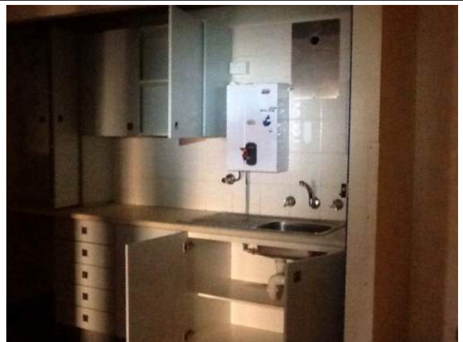
Photo No: J128740-001-MAND-Photo039 Result: SMF - Presumed Positive Building/Level: Main Building-Level One Room/Location: Kitchenette West of Southern Reception Area-West Feature/Material: Boiler Insulation-Insulation Material
