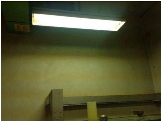
Photo No: J128740-003-HEAL-Photo005 Result: PCB - Presumed Positive Building/Level: Health Services Building-Level One Room/Location: Lift Motor Room-To Ceiling Feature/Material: Fluorescent Light Fitting-Capacitor
