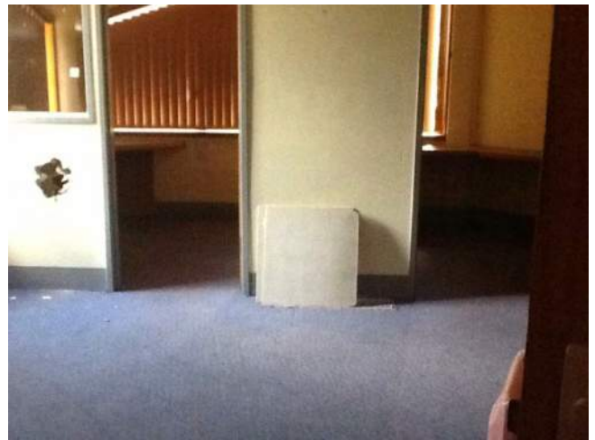
Photo No: J128740-001-MAND-Photo015 Result: Asbestos - Positive Building/Level: Main Building-Level One Room/Location: All areas- Feature/Material: Access Hatch-Fibre Cement Sheetting
