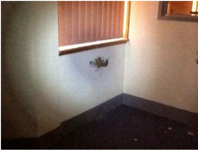
Photo No: J128740-001-MAND-Photo017 Result: SMF - Positive Building/Level: Main Building-Level Two Room/Location: Office Area opposite Tea Room-Wall below Windows Feature/Material: Insulation-Insulation Material
