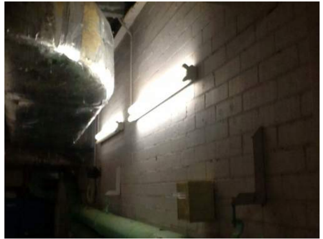
Photo No: J128740-001-MAND-Photo010 Result: PCB - Presumed Positive Building/Level: Main Building-All Levels Room/Location: All areas-Throughout Feature/Material: Fluorescent Light Fitting-Capacitor
