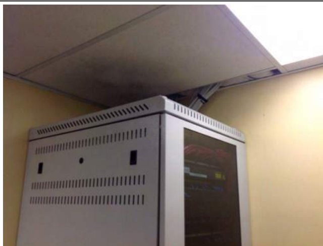
Photo No: J128740-003-HEAL-Photo015 Result: SMF - Presumed Positive Building/Level: Health Services Building-Level One Room/Location: Library Stack Area-West, Above Comms Unit Feature/Material: Penetrations-Pillow Insulation
