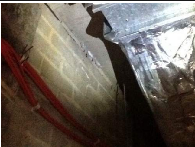
Photo No: J128740-001-MAND-Photo025 Result: Asbestos - Presumed Positive Building/Level: Main Building-Level Two Room/Location: Main Entrance-Adjacent Door Feature/Material: Ceiling Space-Packing
