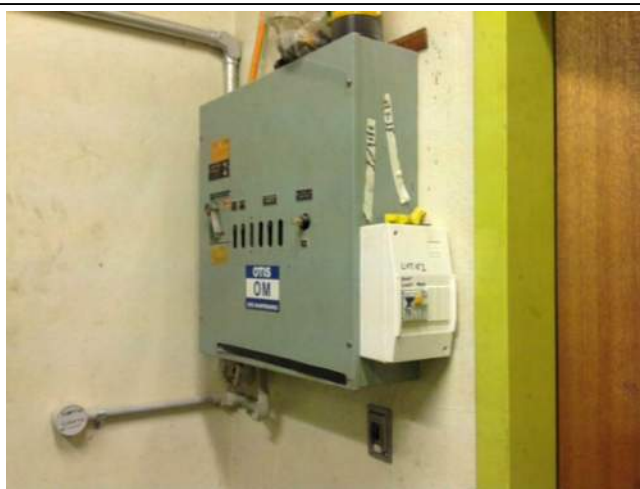
Photo No: J128740-003-HEAL-Photo003 Result: Asbestos - Presumed Positive Building/Level: Health Services Building-Level One Room/Location: Lift Motor Room-East Wall Feature/Material: Electrical Distribution Board-Compressed Bituminous Electrical Panel
