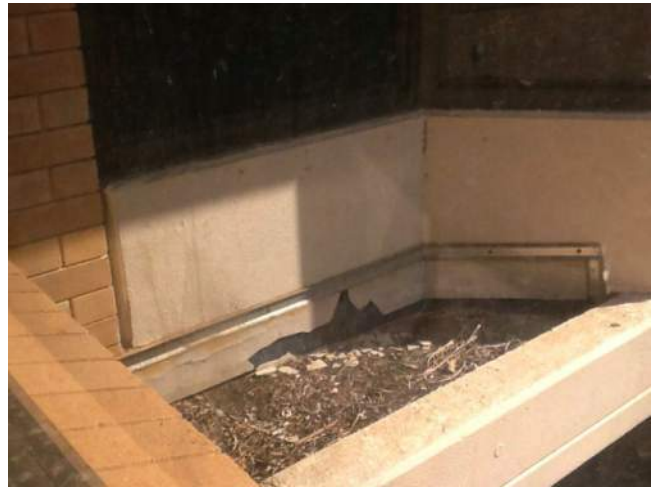
Photo No: J128740-001-MAND-Photo023 Result: Asbestos - Presumed Positive Building/Level: Main Building-Level Two Room/Location: Main Entrance-Adjacent Door Feature/Material: Debris-Fibre Cement Sheetting
