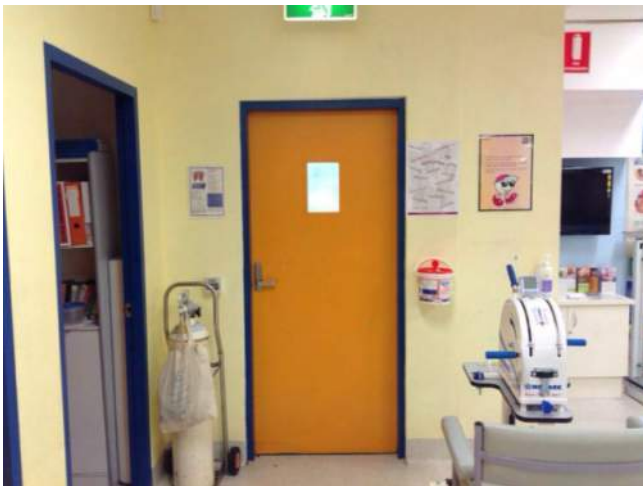
Photo No: J128740-003-HEAL-Photo032 Result: Asbestos - Presumed Positive Building/Level: Health Services Building-Level Two Room/Location: Physio and OT Treatment Area-Northwest Feature/Material: Fire Door-Fire Door Core
