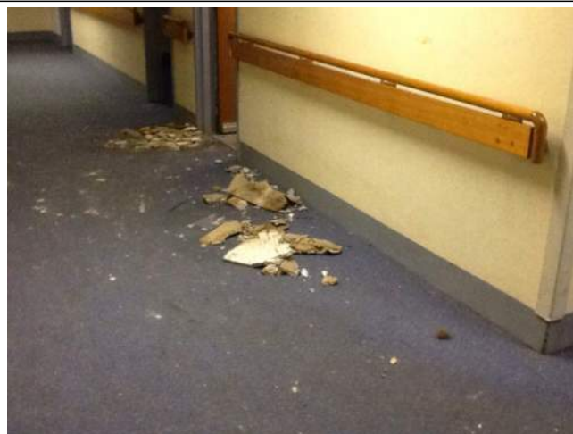
Photo No: J128740-001-MAND-Photo012 Result: SMF - Positive Building/Level: Main Building-Levels One & Two Room/Location: Various Rooms-Throughout Feature/Material: On Ground-Compressed Ceiling Tiles
