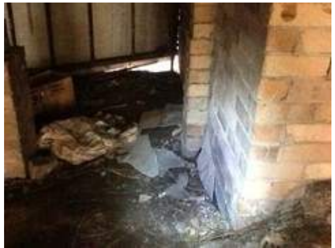
Photo No: J128740-002-ABOR-Photo101 Result: Asbestos - Presumed Positive Building/Level: Main Building-All Levels Room/Location: Various Throughout-Throughout Feature/Material: Debris-Fibre Cement Sheetting
