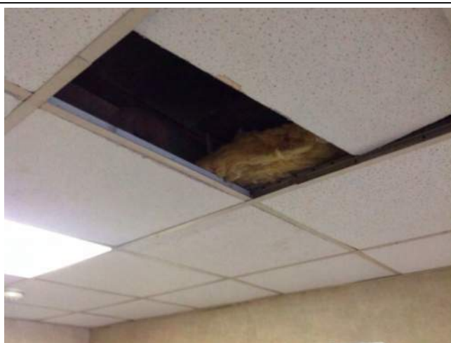
Photo No: J128740-003-HEAL-Photo041 Result: SMF - Presumed Positive Building/Level: Health Services Building-Level Three Room/Location: Main Corridor-Ceiling Space Feature/Material: Insulation Batts-Insulation Material
