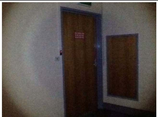
Photo No: J128740-001-MAND-Photo019 Result: Asbestos - Presumed Positive Building/Level: Main Building-Level Two Room/Location: Northern Fire Stairwell-Entrance Feature/Material: Fire Door-Fire Door Core
