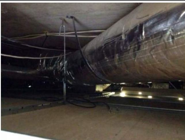
Photo No: J128740-003-HEAL-Photo046 Result: SMF - Presumed Positive Building/Level: Health Services Building-Level Two Room/Location: Throughout Level-Ceiling Space Feature/Material: Flexible Ductwork Insulation-Insulation Material
