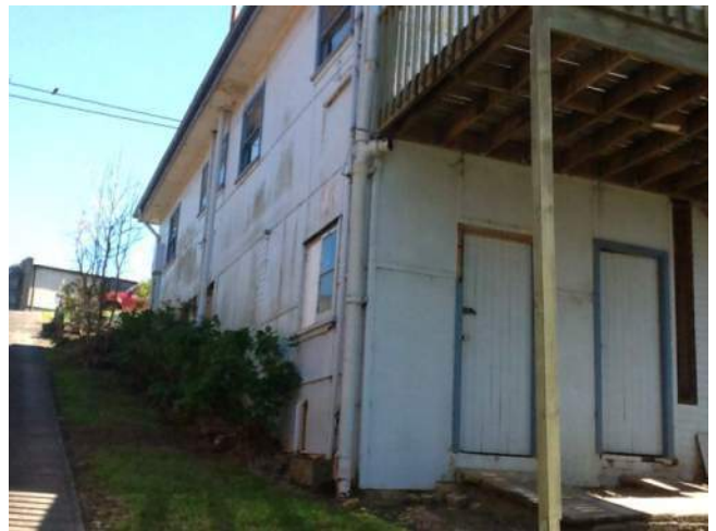
Photo No: J128740-002-ABOR-Photo001 Result: Asbestos - Positive Building/Level: Main Building-Ground Level Room/Location: Surroundings-Throughout Feature/Material: Wall-Fibre Cement Sheetting
