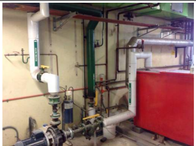
Photo No: J128740-003-HEAL-Photo009 Result: SMF - Presumed Positive Building/Level: Health Services Building-Level One Room/Location: Plant Room-From Boiler Feature/Material: Pipework Insulation-Insulation Material
