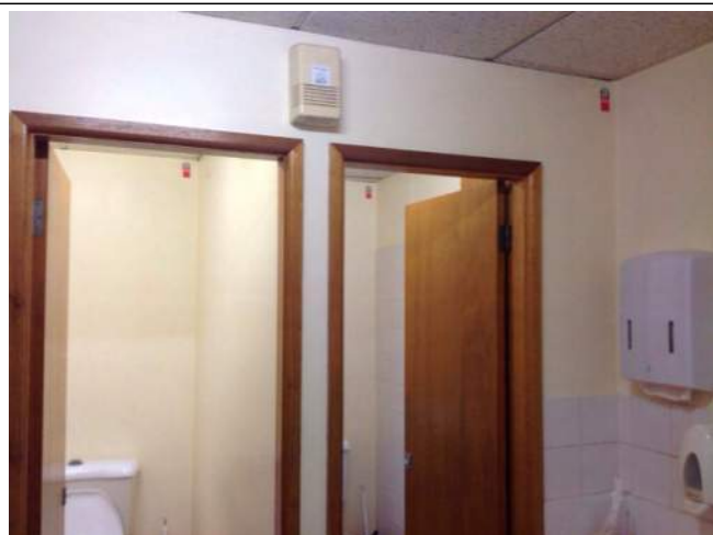
Photo No: J128740-003-HEAL-Photo027 Result: Asbestos - Previously Sampled Positive Building/Level: Health Services Building-Level Three Room/Location: Female Toilets-Throughout Feature/Material: Wall-Fibre Cement Sheetting
