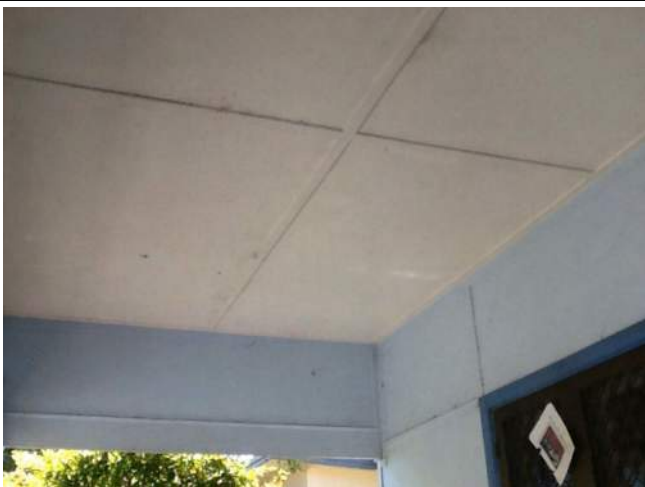
Photo No: J128740-002-ABOR-Photo013 Result: Asbestos - Presumed Positive Building/Level: Main Building-Ground Level Room/Location: Front Porch-Throughout Feature/Material: Ceiling-Fibre Cement Sheetting
