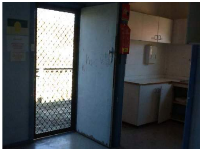
Photo No: J128740-002-ABOR-Photo010 Result: Lead (Paint) - Positive Building/Level: Main Building-Ground Level Room/Location: Back Entrance- Feature/Material: Door-Paint System/s
