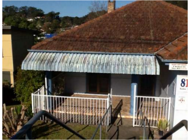
Photo No: J128740-002-ABOR-Photo022 Result: Lead (Paint) - Presumed Positive Building/Level: Main Building-Ground Level Room/Location: Front Porch- Feature/Material: Awning-Paint System/s
