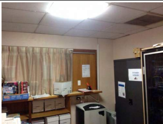
Photo No: J128740-003-HEAL-Photo018 Result: SMF - Presumed Positive Building/Level: Health Services Building-Level Three Room/Location: Human Resources-Photocopy Room Feature/Material: Ceiling Tiles-Insulation Material
