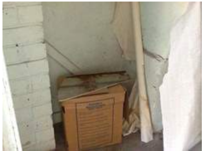
Photo No: J128740-002-ABOR-Photo100 Result: Asbestos - Presumed Positive Building/Level: Main Building-Basement Room/Location: Laundry (adjacent Toilets)-Along Southern Wall Feature/Material: On Ground-Fibre Cement Debris
