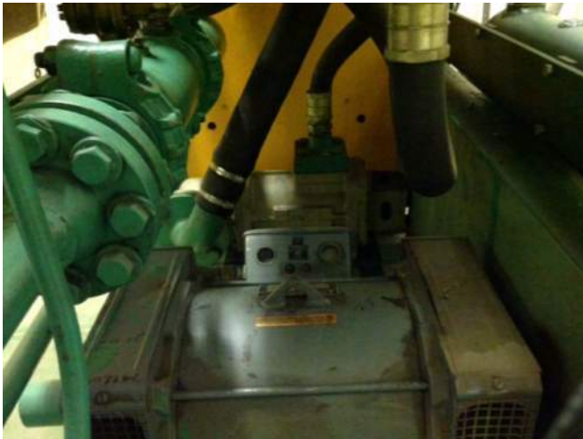
Photo No: J128740-003-HEAL-Photo006 Result: Asbestos - Presumed Positive Building/Level: Health Services Building-Level One Room/Location: Lift Motor Room-Hydraulic Lift Motor Feature/Material: Pipework Flange Joint-Gasket Material
