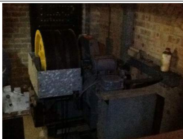
Photo No: J128740-001-MAND-Photo001 Result: Asbestos - Presumed Positive Building/Level: Main Building-Level Three Room/Location: Lift Motor Room- Feature/Material: Lift Motor-Brake Pads
