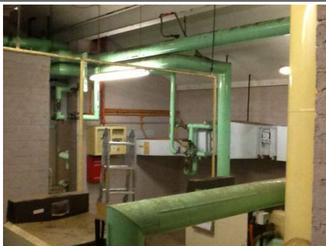
Photo No: J128740-001-MAND-Photo003 Result: SMF - Presumed Positive Building/Level: Main Building-Level Three Room/Location: All areas-Throughout Feature/Material: Pipework Insulation-Insulation Material
