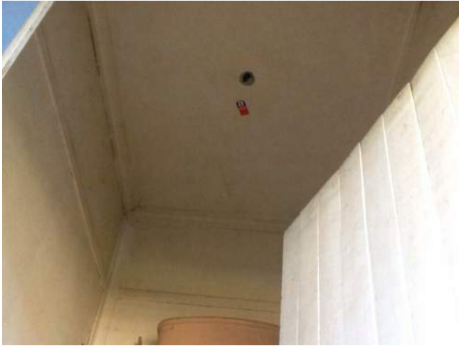
Photo No: J128740-002-ABOR-Photo019 Result: Asbestos - Presumed Positive Building/Level: Main Building-Basement Room/Location: Toilets & Laundry-Throughout Feature/Material: Ceiling-Fibre Cement Sheetting
