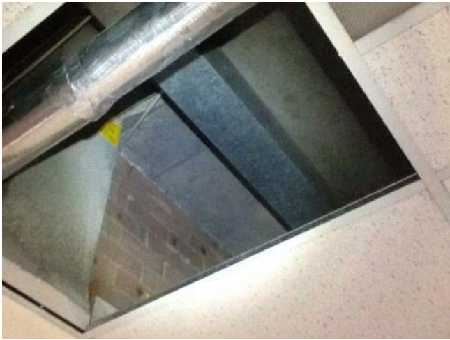
Photo No: J128740-001-MAND-Photo038 Result: SMF - Positive Building/Level: Main Building-Level One Room/Location: Room 5 (adjacent Kitchen)-Northeast Feature/Material: Ceiling-Kao-Wool
