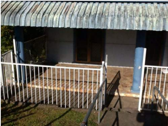
Photo No: J128740-002-ABOR-Photo021 Result: Lead (Paint) - Presumed Positive Building/Level: Main Building-Ground Level Room/Location: Front Porch- Feature/Material: Beam-Paint System/s
