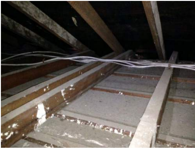
Photo No: J128740-002-ABOR-Photo006 Result: Lead (Dust) - Positive Building/Level: Main Building-Ground Level Room/Location: Roof Space-Throughout Feature/Material: All surfaces-Accumulated Dust
