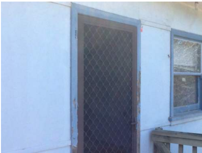
Photo No: J128740-002-ABOR-Photo009 Result: Lead (Paint) - Positive Building/Level: Main Building-Ground Level Room/Location: All rooms-Throughout Feature/Material: Windows & Door Frames-Paint System/s
