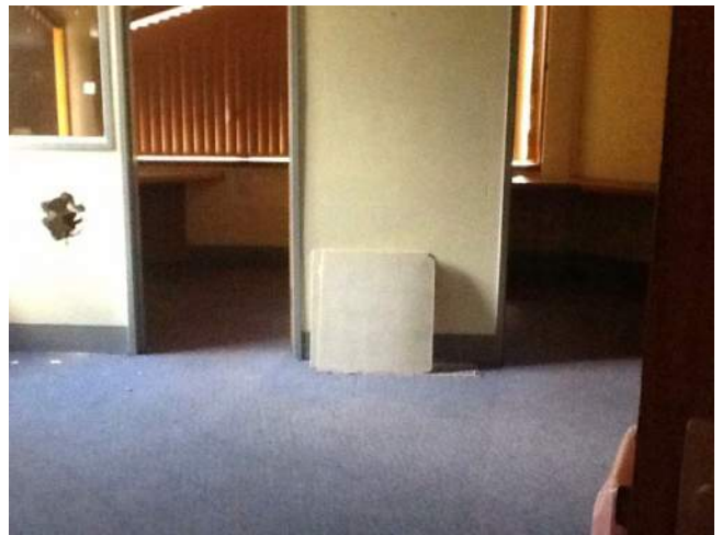
Photo No: J128740-001-MAND-Photo015 Result: Asbestos - Presumed Positive Building/Level: Main Building-Level Two Room/Location: All areas- Feature/Material: Access Hatch-Fibre Cement Sheetting
