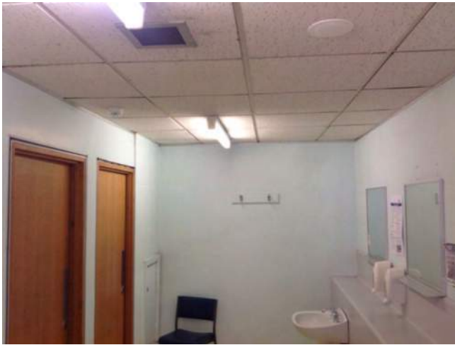
Photo No: J128740-003-HEAL-Photo034 Result: SMF - Presumed Positive Building/Level: Health Services Building-Level One Room/Location: Women's Health, Nurses Clinic and Toilets-Throughout Feature/Material: Ceiling Tiles-Insulation Material
