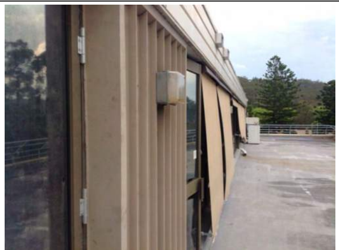
Photo No: J128740-003-HEAL-Photo029 Result: Asbestos - Previously Sampled Positive Building/Level: Health Services Building-Level Three Room/Location: Surrounding- Feature/Material: Eaves-Fibre Cement Sheetting
