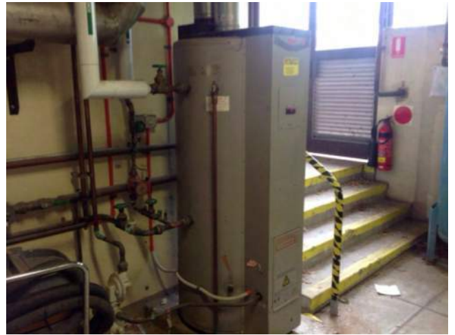
Photo No: J128740-003-HEAL-Photo010 Result: SMF - Presumed Positive Building/Level: Health Services Building-Level One Room/Location: Plant Room-Southeast Feature/Material: Hot Water Heater-Insulation Material
