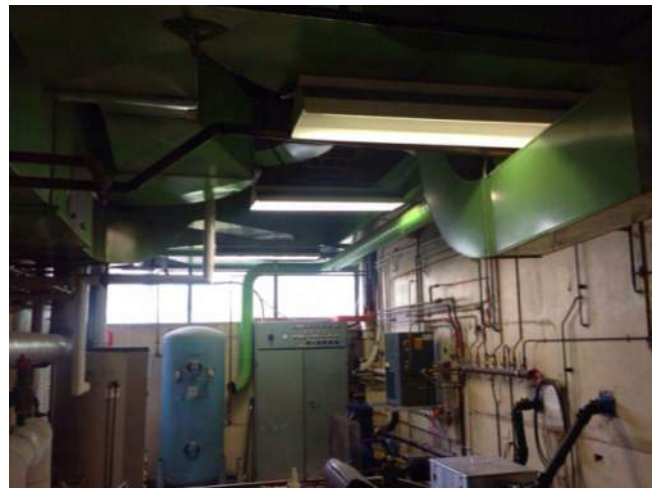
Photo No: J128740-003-HEAL-Photo013 Result: PCB - Presumed Positive Building/Level: Health Services Building-Level One Room/Location: Plant Room-Throughout Feature/Material: Fluorescent Light Fitting-Capacitor
