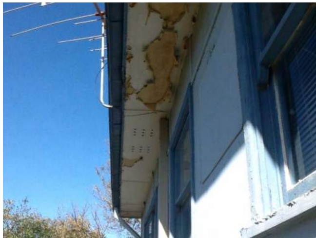
Photo No: J128740-002-ABOR-Photo015 Result: Asbestos - Presumed Positive Building/Level: Main Building-Ground Level Room/Location: Surroundings-Throughout Feature/Material: Eaves-Fibre Cement Sheetting
