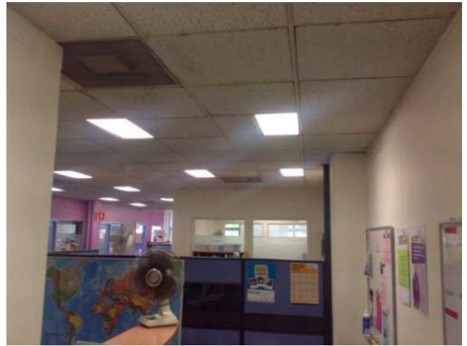
Photo No: J128740-003-HEAL-Photo033 Result: SMF - Presumed Positive Building/Level: Health Services Building-Level Two Room/Location: Mid-Southern Offices-Throughout Feature/Material: Ceiling Tiles-Insulation Material
