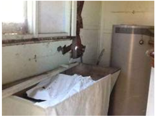
Photo No: J128740-002-ABOR-Photo103 Result: Asbestos - Positive Building/Level: Main Building-Basement Room/Location: All rooms-Throughout Feature/Material: Wall-Fibre Cement Sheetting
