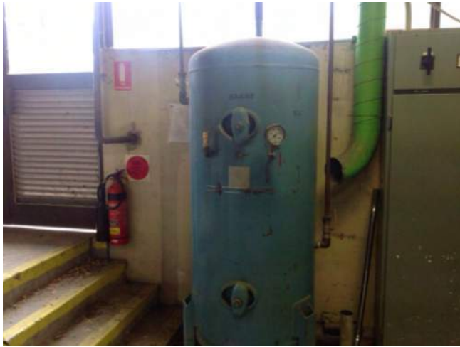
Photo No: J128740-003-HEAL-Photo012 Result: Asbestos - Presumed Positive Building/Level: Health Services Building-Level One Room/Location: Plant Room-South Feature/Material: Boiler-Insulation
