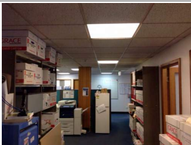
Photo No: J128740-003-HEAL-Photo022 Result: SMF - Presumed Positive Building/Level: Health Services Building-Level Three Room/Location: Finance Offices including Toilet-Throughout Feature/Material: Ceiling Tiles-Insulation Material
