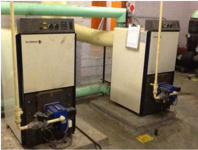
Photo No: J128740-001-MAND-Photo009 Result: SMF - Presumed Positive Building/Level: Main Building-Level Three Room/Location: Plant Room- Feature/Material: Boiler Insulation-Insulation Material
