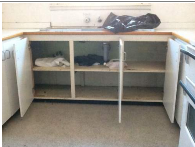
Photo No: J128740-002-ABOR-Photo004 Result: Asbestos - Presumed Positive Building/Level: Main Building-Ground Level Room/Location: Kitchen-Throughout Feature/Material: Infill Panels - Low Level-Fibre Cement Sheetting
