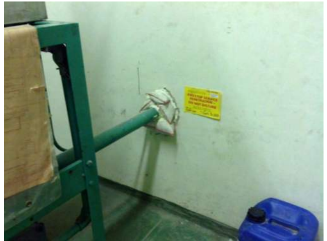
Photo No: J128740-003-HEAL-Photo004 Result: SMF - Presumed Positive Building/Level: Health Services Building-Level One Room/Location: Lift Motor Room-Northern Side Feature/Material: Penetrations-Pillow Insulation
