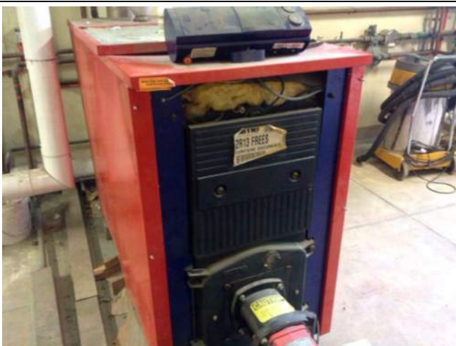
Photo No: J128740-003-HEAL-Photo008 Result: SMF - Presumed Positive Building/Level: Health Services Building-Level One Room/Location: Plant Room- Feature/Material: Boiler Insulation-Insulation Material
