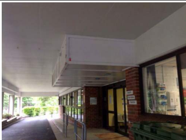
Photo No: J128740-003-HEAL-Photo028 Result: Asbestos - Previously Sampled Positive Building/Level: Health Services Building-Level One Room/Location: South-West Entrance-Ceiling Feature/Material: Awning-Fibre Cement Sheetting
