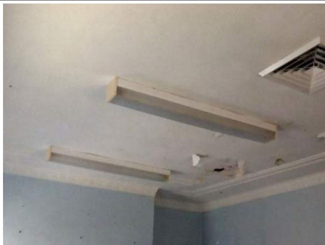
Photo No: J128740-002-ABOR-Photo011 Result: PCB - Presumed Positive Building/Level: Main Building-Ground Level Room/Location: All rooms- Feature/Material: Fluorescent Light Fitting - Double Tube-Capacitor
