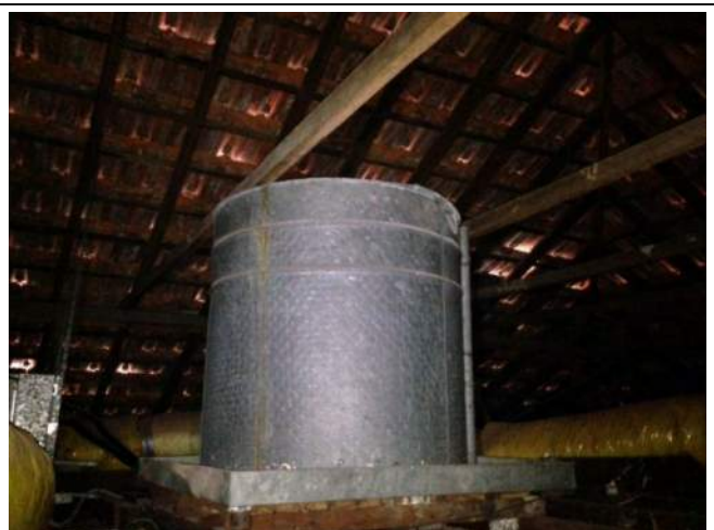
Photo No: J128740-002-ABOR-Photo007 Result: Asbestos - Presumed Positive Building/Level: Main Building-Ground Level Room/Location: Roof Space-Central Feature/Material: Storage Tank-Insulation
