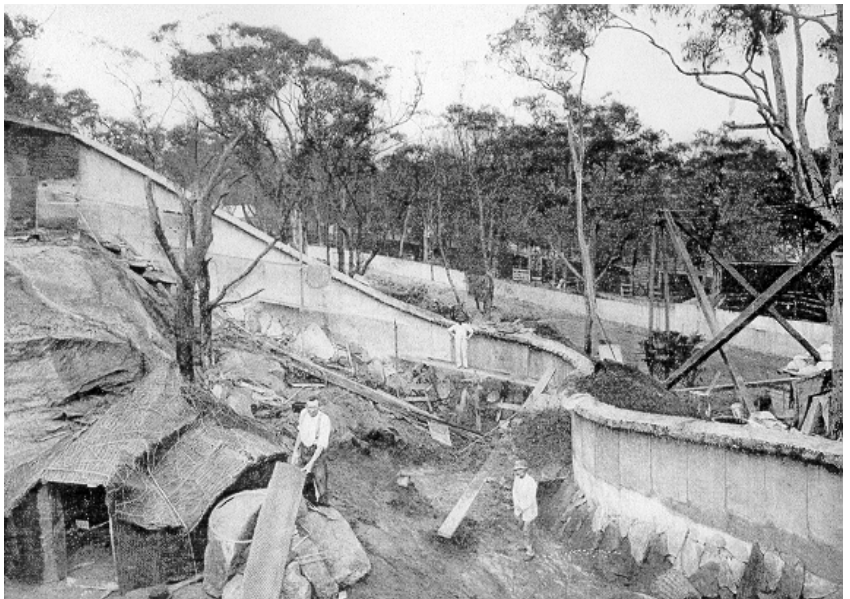
Figure 3.5 The construction of one of the circular monkey pits, c1915. Note the natural bushland in the background (Taronga Zoo Archives).
