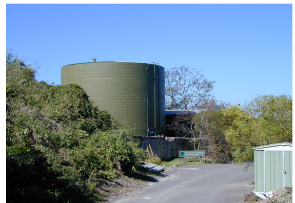
Figure 7.10 The Waste Water Treatment Plant that services the Zoo.
