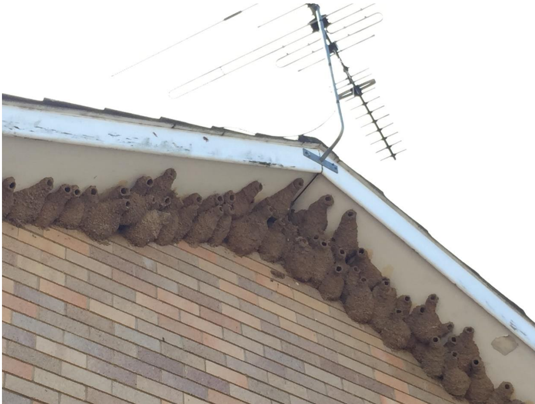
Plate 2. Accumulation of active and disused Fairy Martin ( Petrochelidon ariel ) bird nests recorded by Land Eco Consulting on the Subject Land. Bats are known to utilise this type of bird nest as roost habitat.
