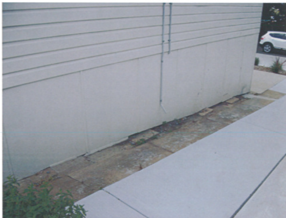
Photograph 4: Possible ACM sheeting on western wall of 61 Uralba Street
