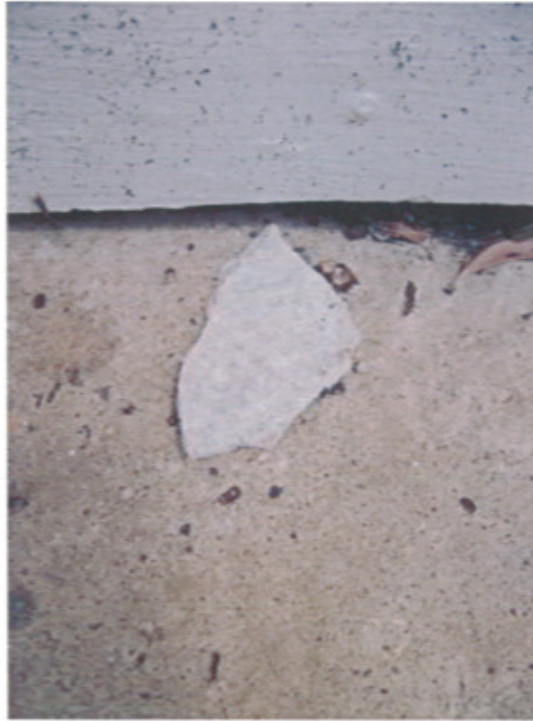
Photograph 5: PACM sheeting fragment
