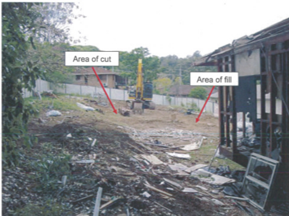
Photograph 20: View east from the western boundary of 26 Dalziell Street and areas of cut/fill activities to form a level platform for the buildings
