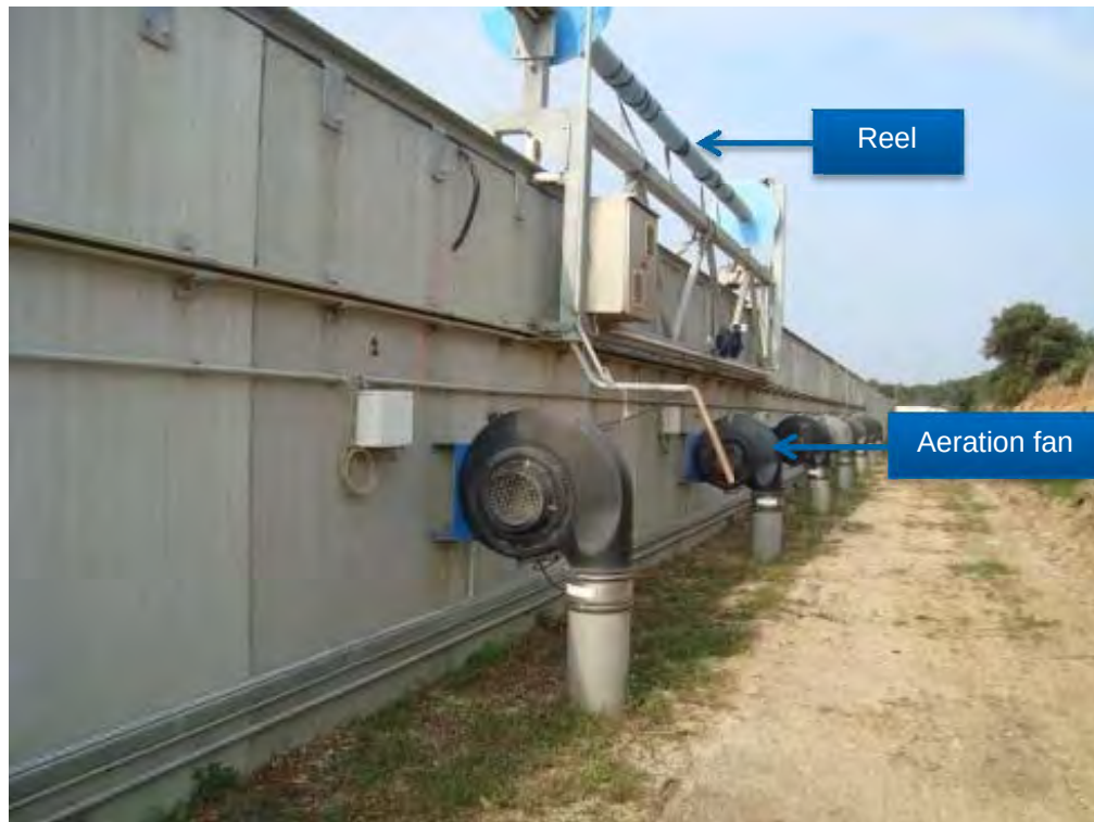
Photo 6.2 Example of bunker aeration and cover system infrastructure
