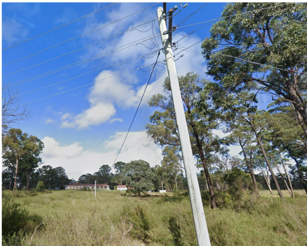
Image 4 – Existing Low Voltage Overhead Powerline Extension to Customer Pole to Serve the Existing Residence.
