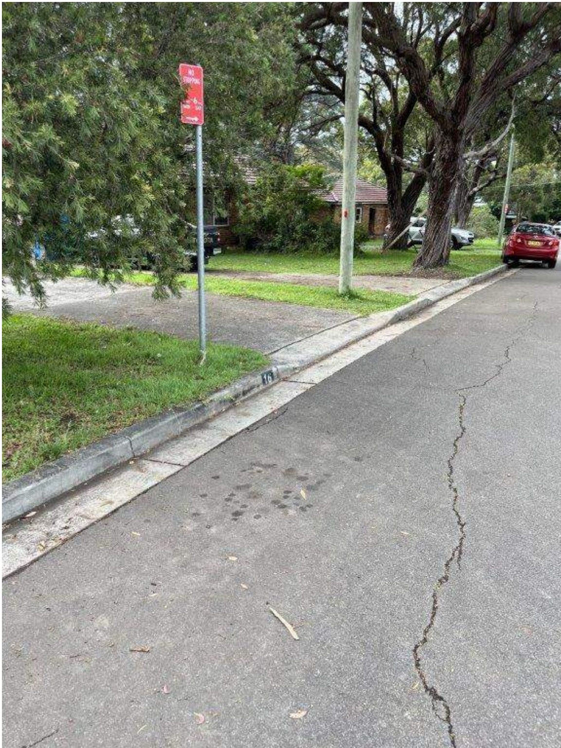
Photo 84 - Hinkler Avenue - Cracking of pavement
