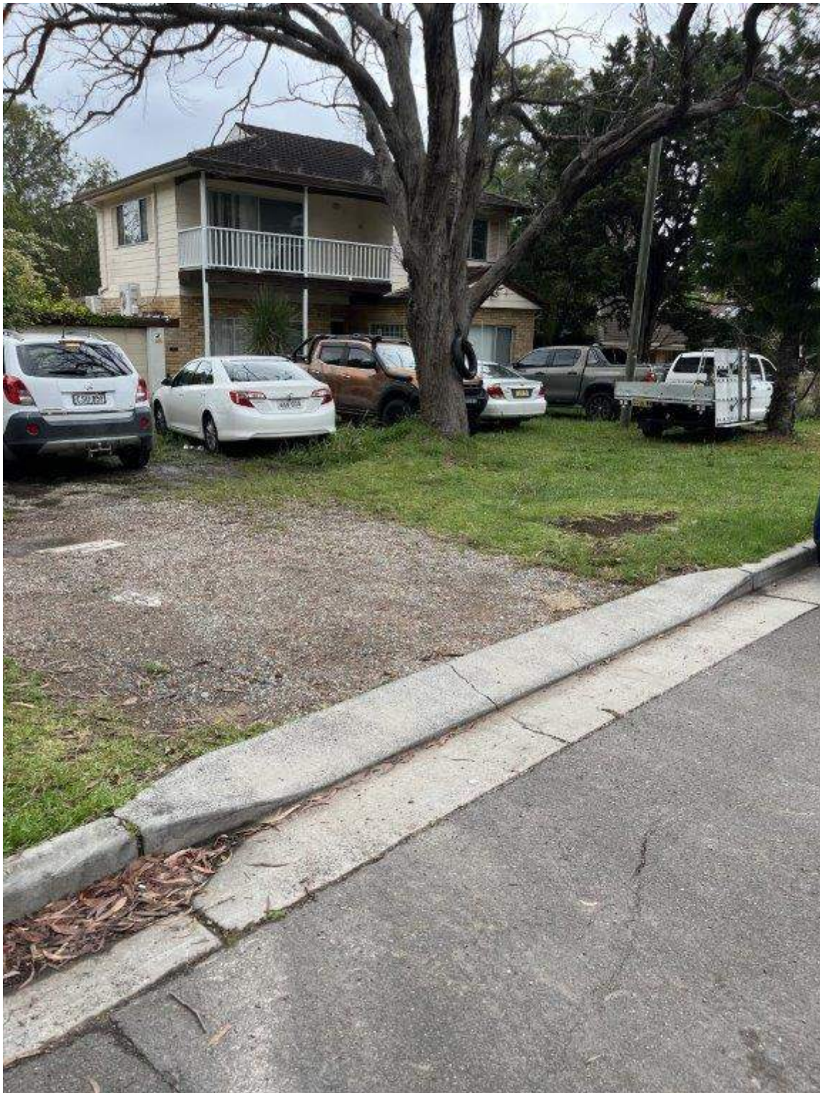
Photo 39 - Hinkler Avenue - Cracking of pavement
