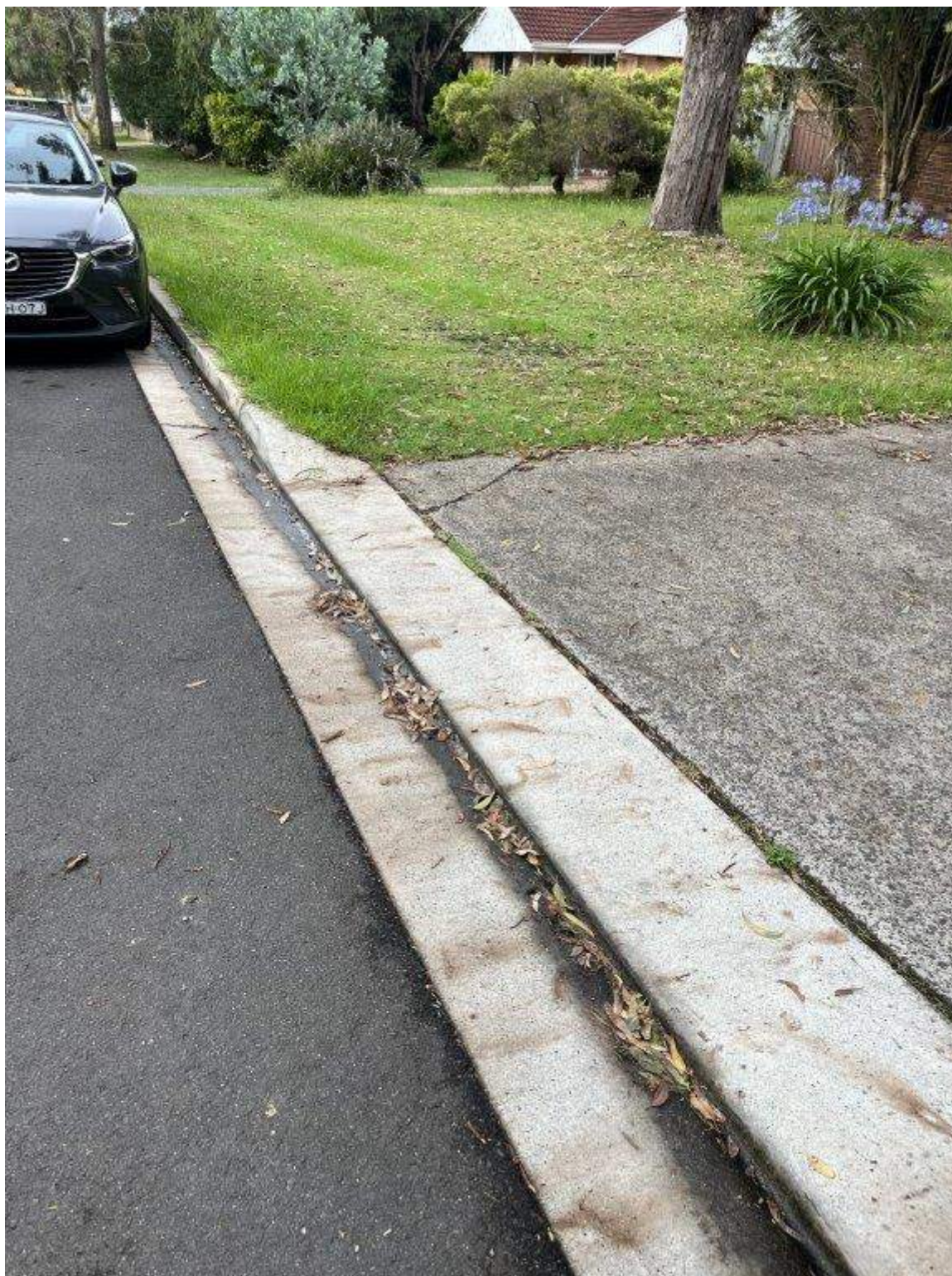
Photo 194 - Taren Point Road - Cracking of pavement
