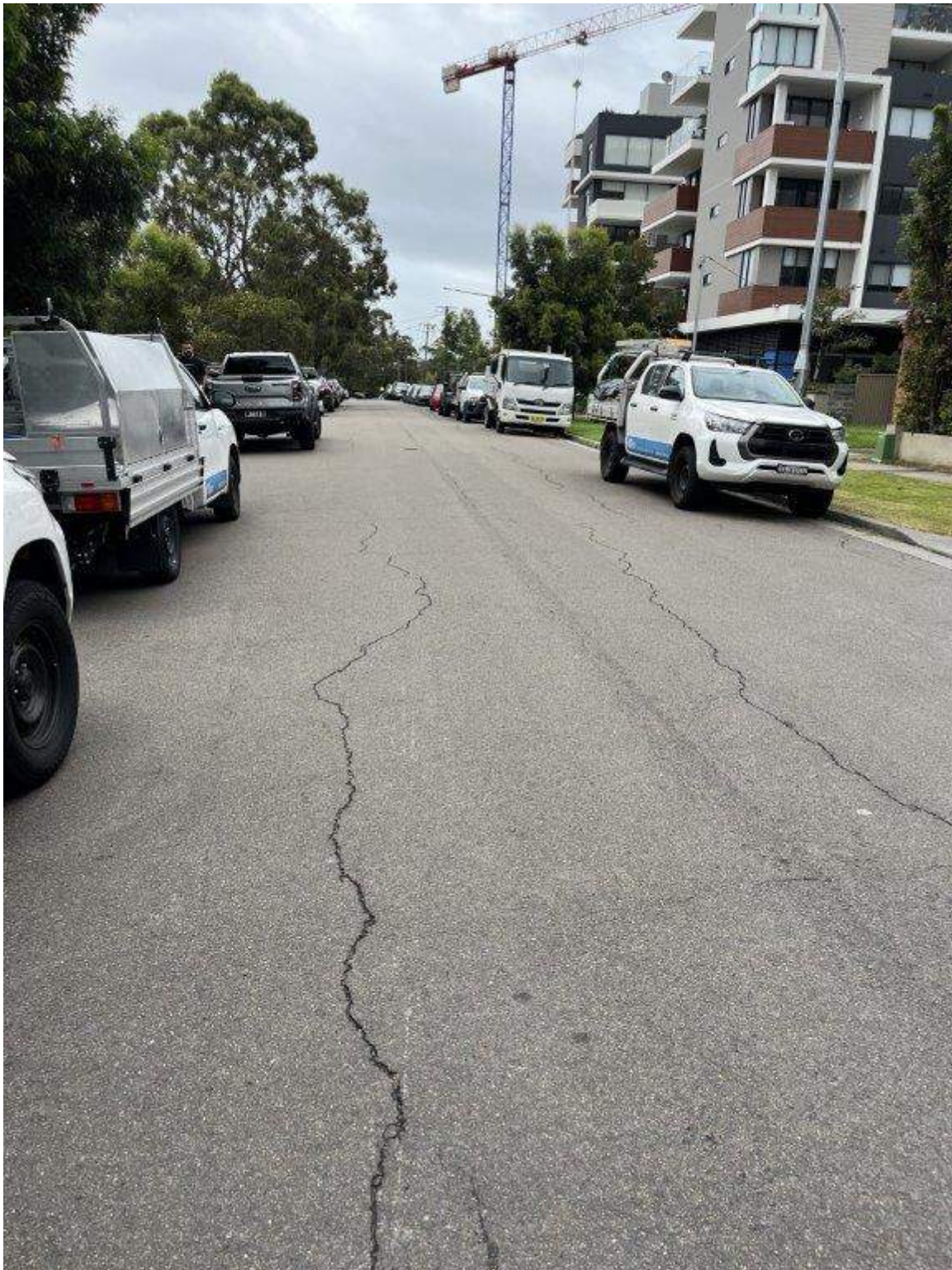
Photo 10 - Hinkler Avenue - Cracking of pavement
