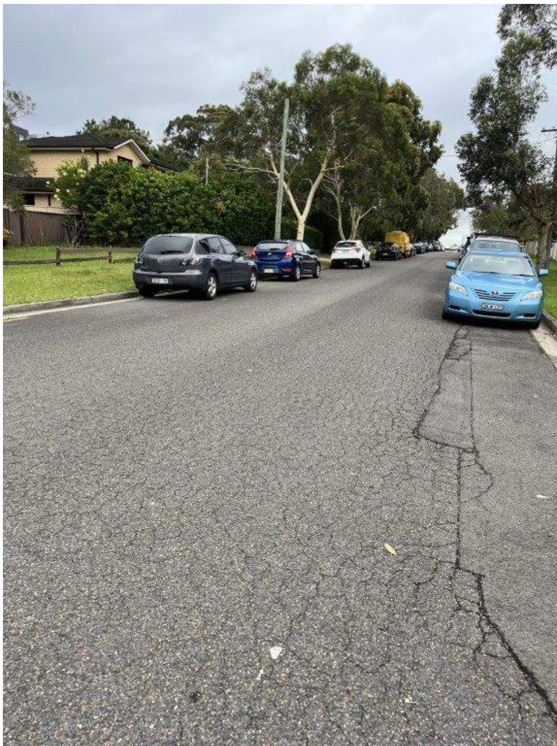
Photo 147 - Taren Point Road - Cracking of pavement
