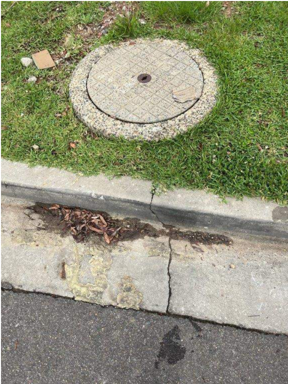
Photo 79 - Hinkler Avenue - Cracking of kerb and pavement
