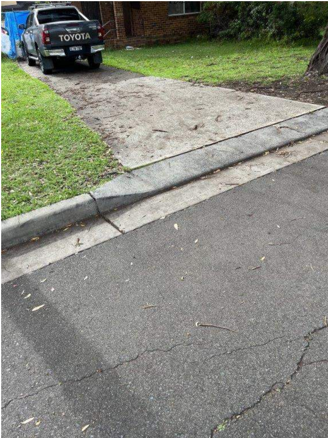
Photo 92 - Hinkler Avenue - Cracking of pavement
