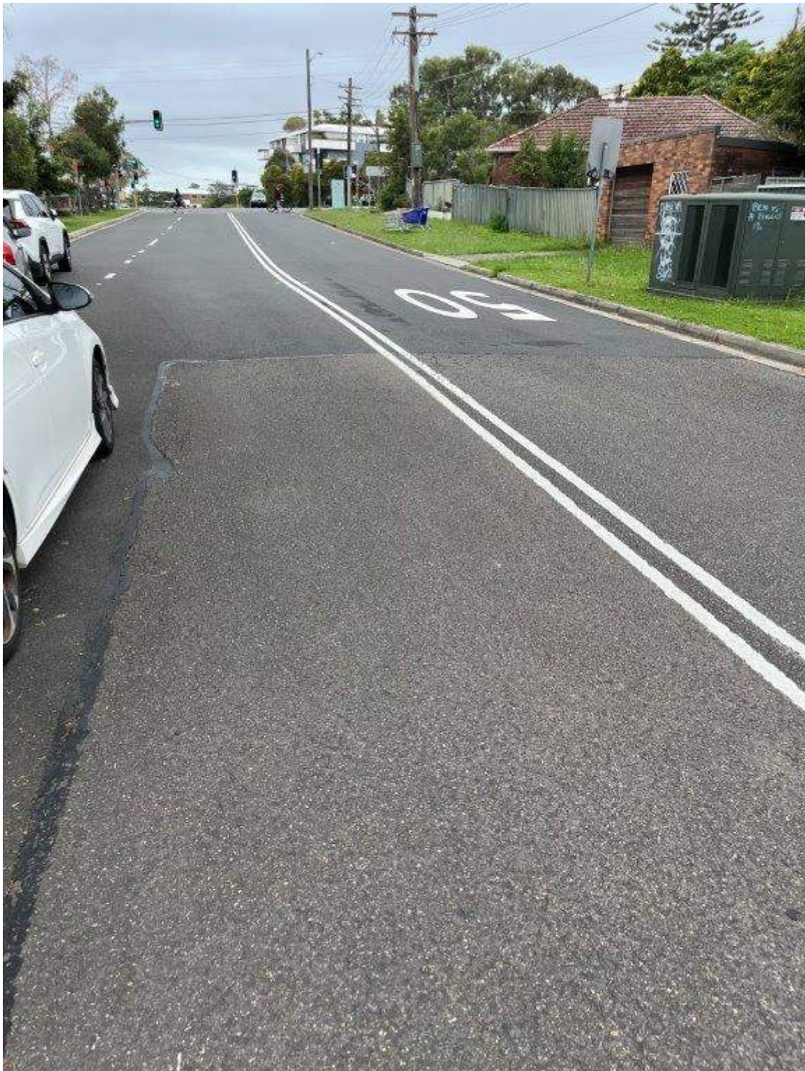
Photo 221 - Taren Point Road - Existing condition of pavement
