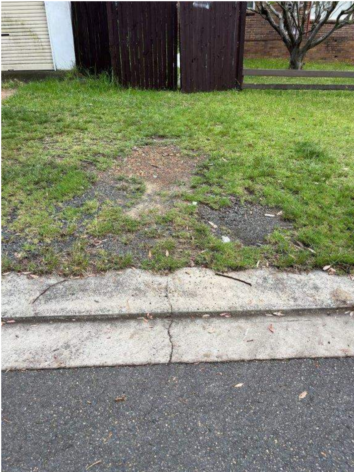
Photo 134 - Hinkler Avenue - Cracking of pavement
