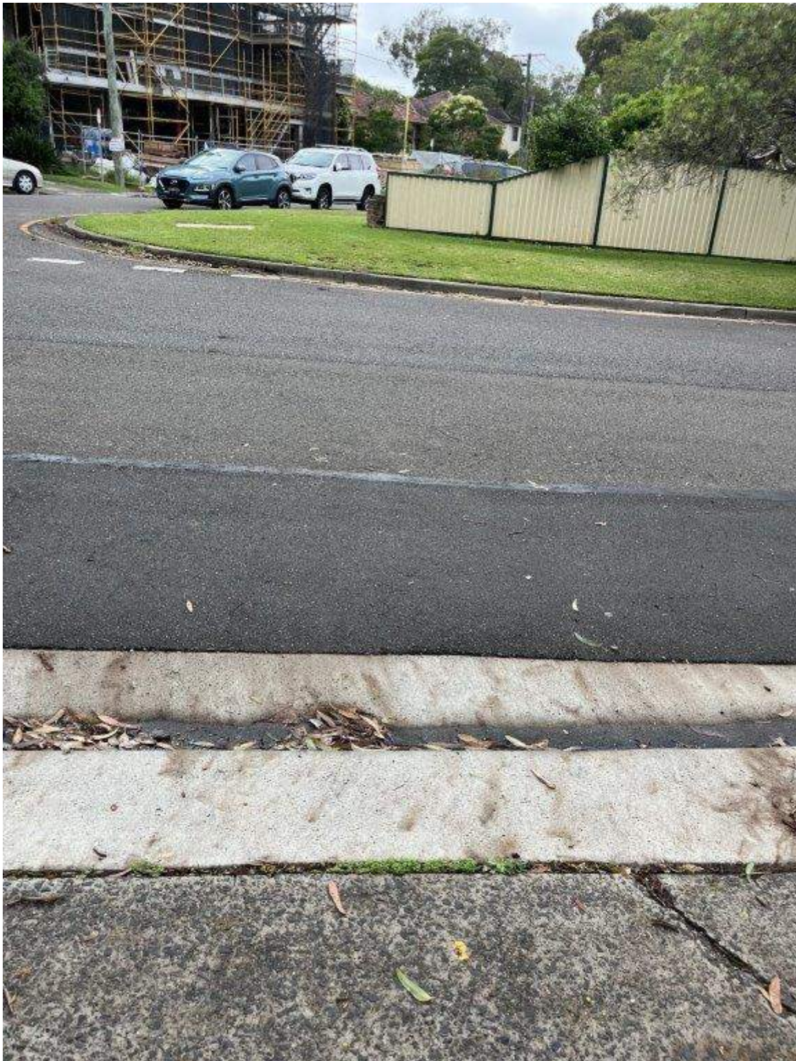
Photo 196 - Taren Point Road - Cracking of pavement
