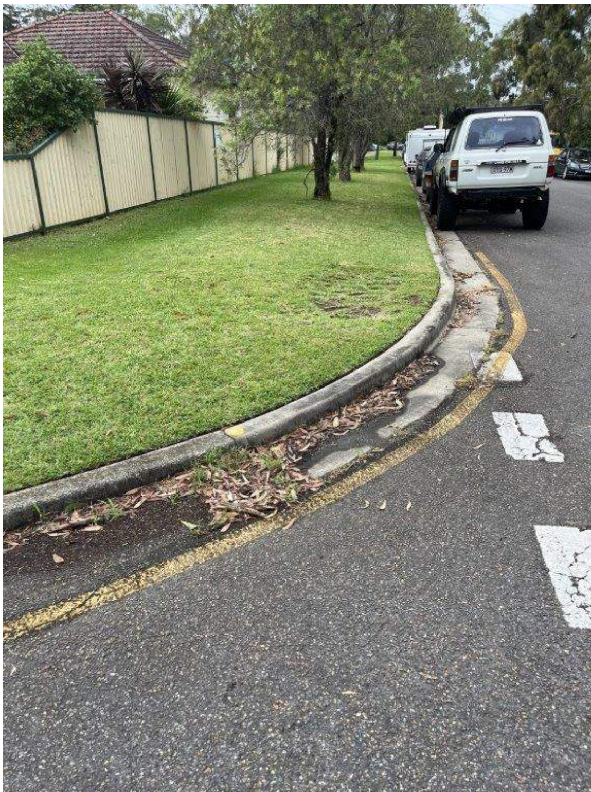
Photo 191 - Taren Point Road - Cracking of pavement
