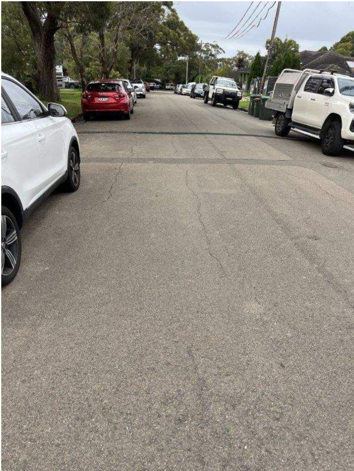
Photo 66 - Hinkler Avenue - Cracking of pavement
