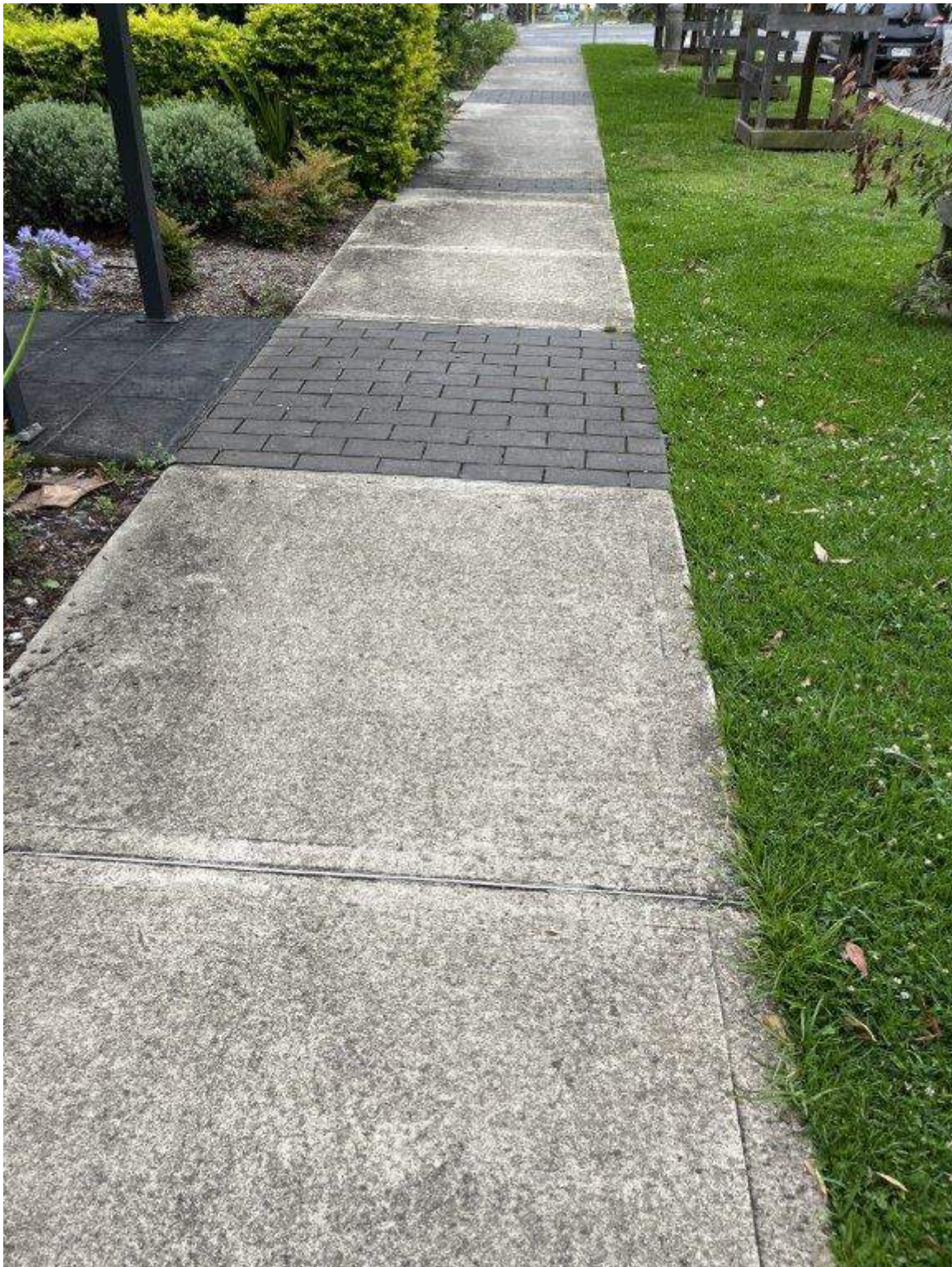
Photo 258 - Taren Point Road - Existing condition of pavement
