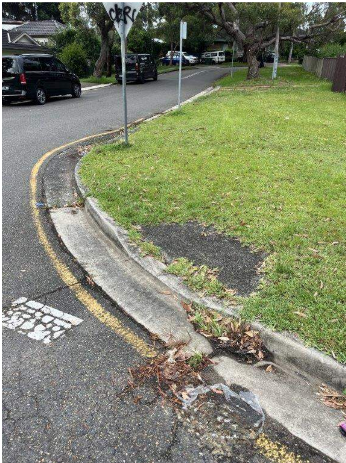
Photo 149 - Taren Point Road - Cracking of pavement
