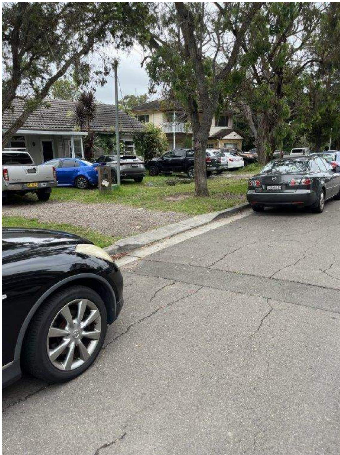
Photo 32 - Hinkler Avenue - Cracking of pavement
