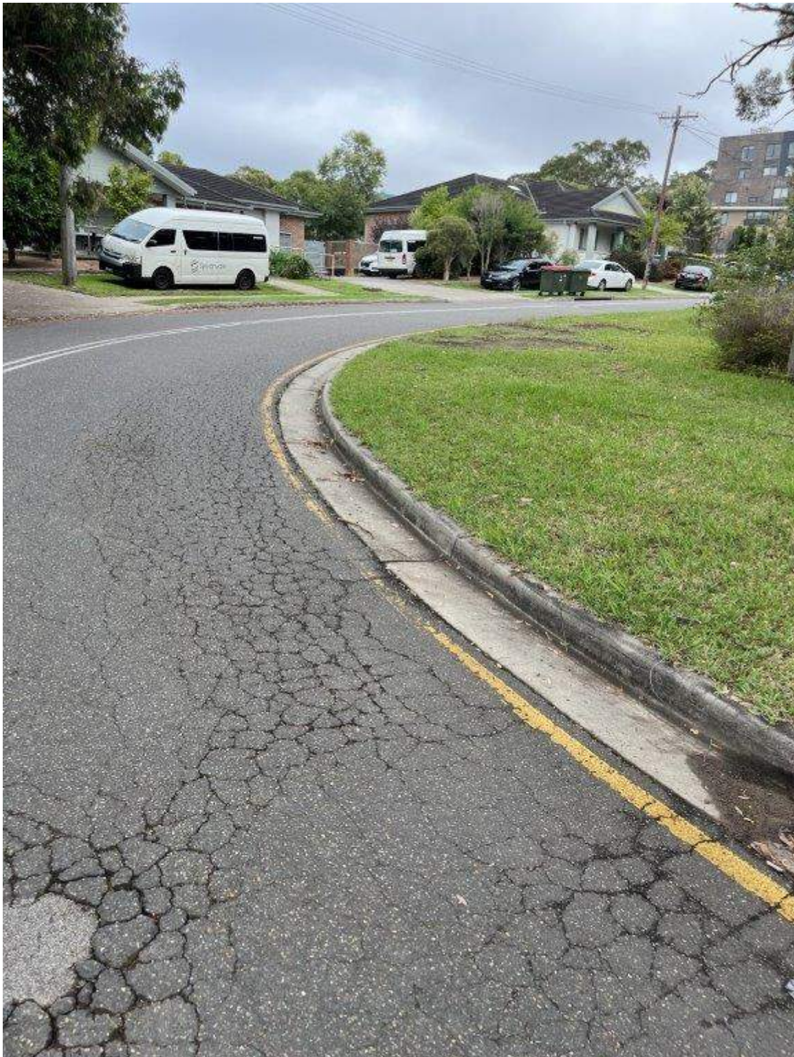
Photo 122 - Hinkler Avenue - Cracking of pavement
