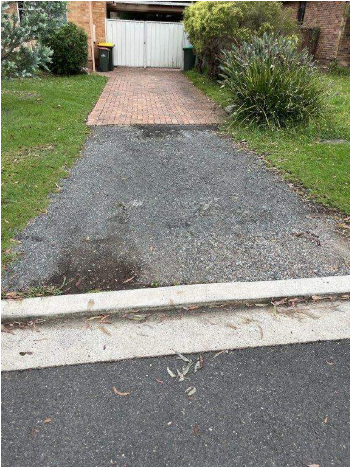
Photo 183 - Taren Point Road - Existing condition of pavement
