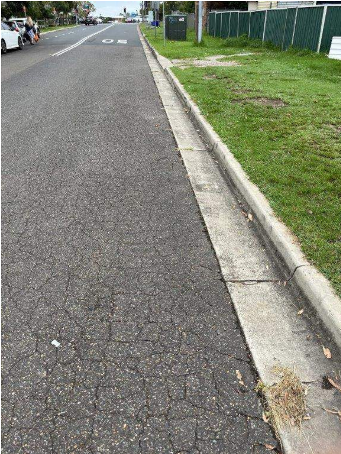
Photo 214 - Taren Point Road - Cracking of pavement
