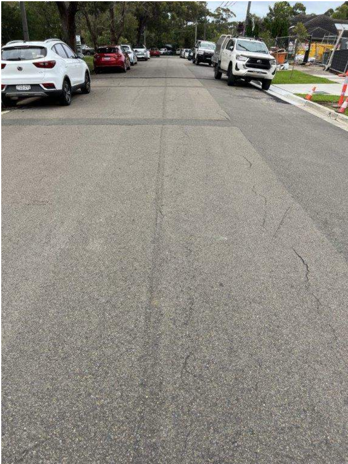
Photo 61 - Hinkler Avenue - Cracking of pavement
