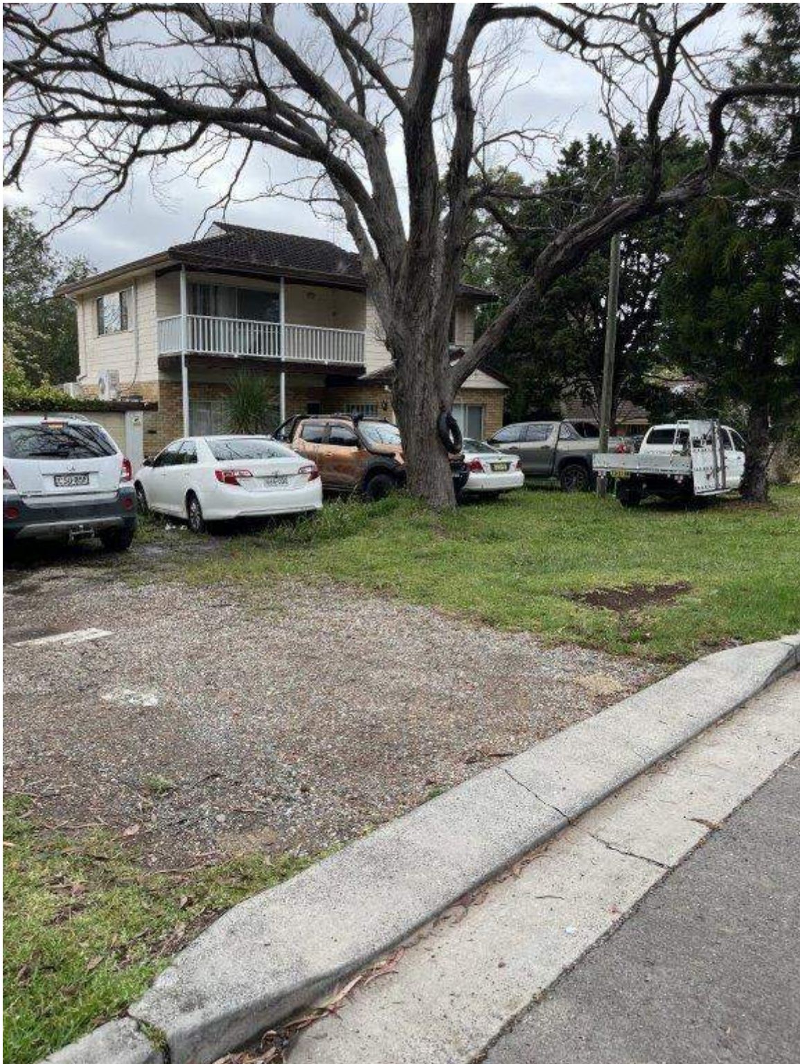
Photo 52 - Hinkler Avenue - Cracking of pavement
