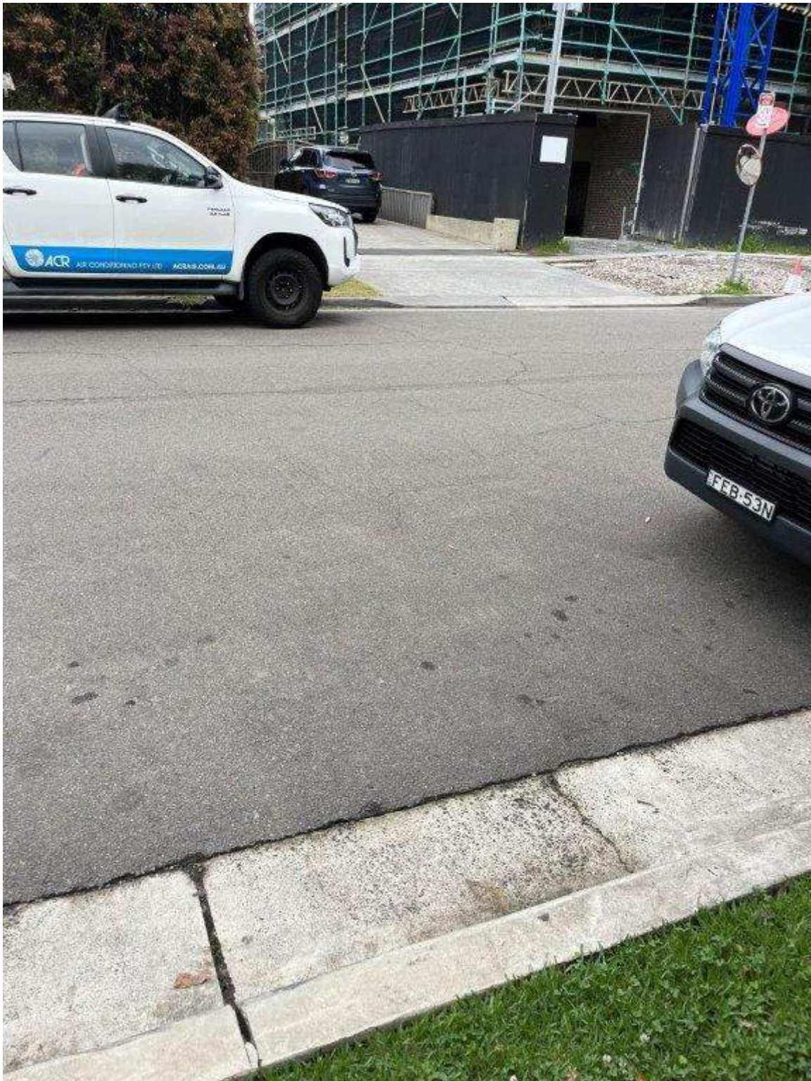
Photo 15 - Hinkler Avenue - Cracking of pavement
