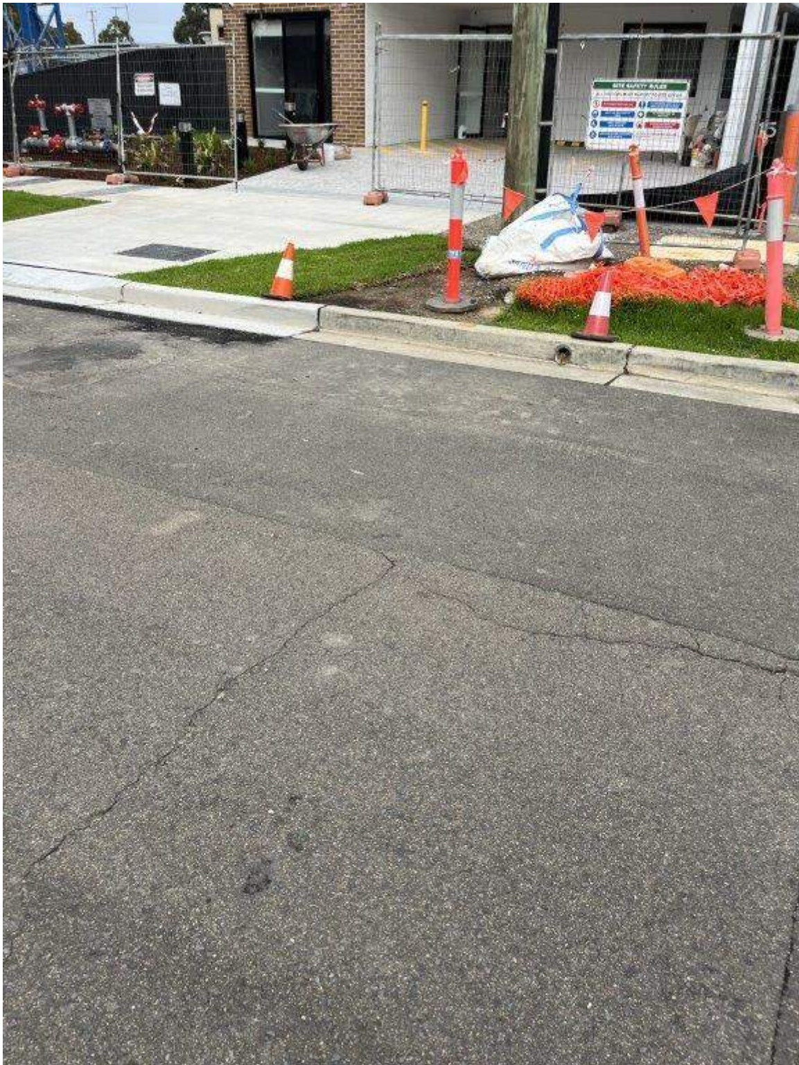
Photo 67 - Hinkler Avenue - Cracking of pavement
