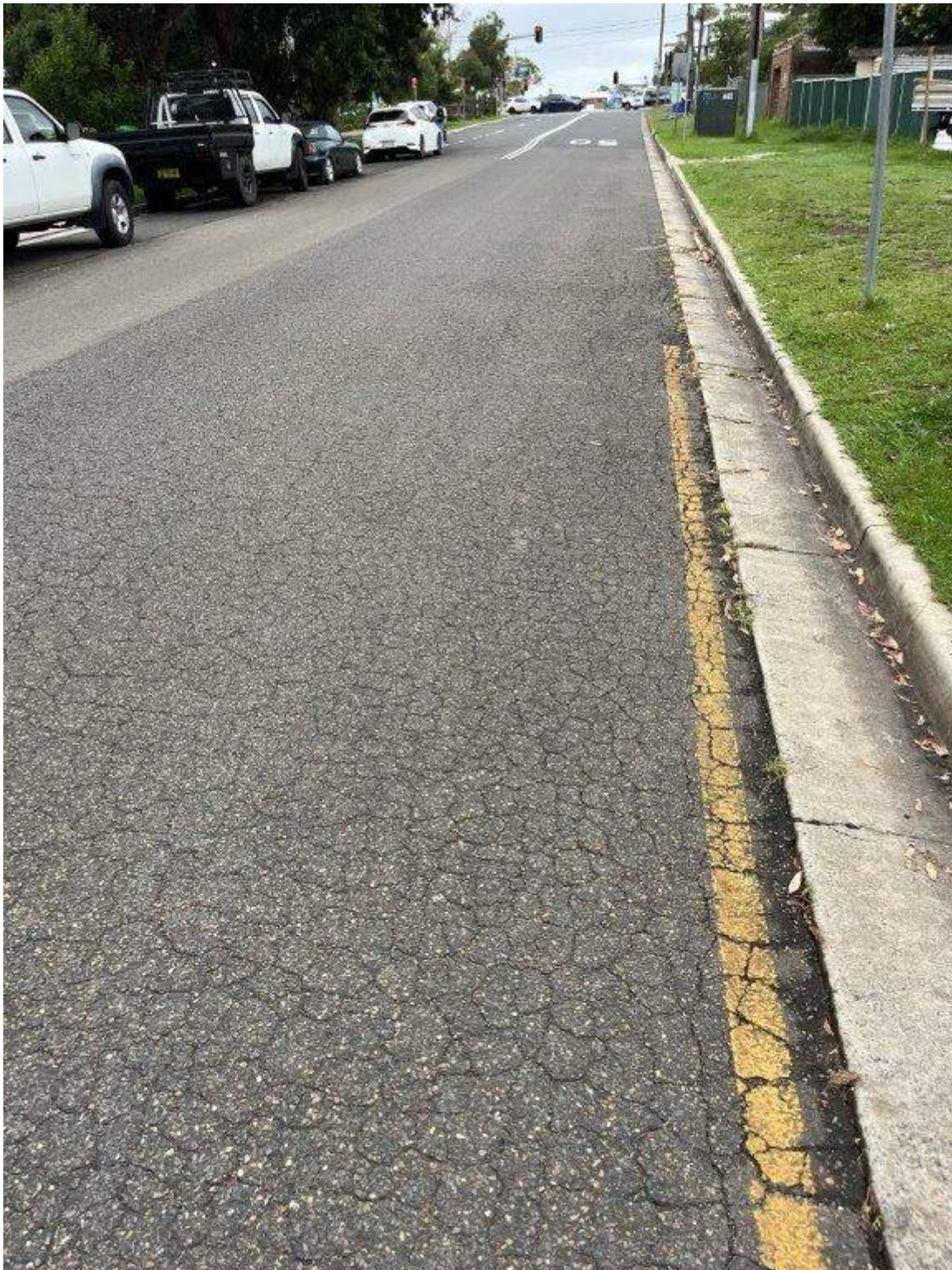
Photo 207 - Taren Point Road - Cracking of pavement
