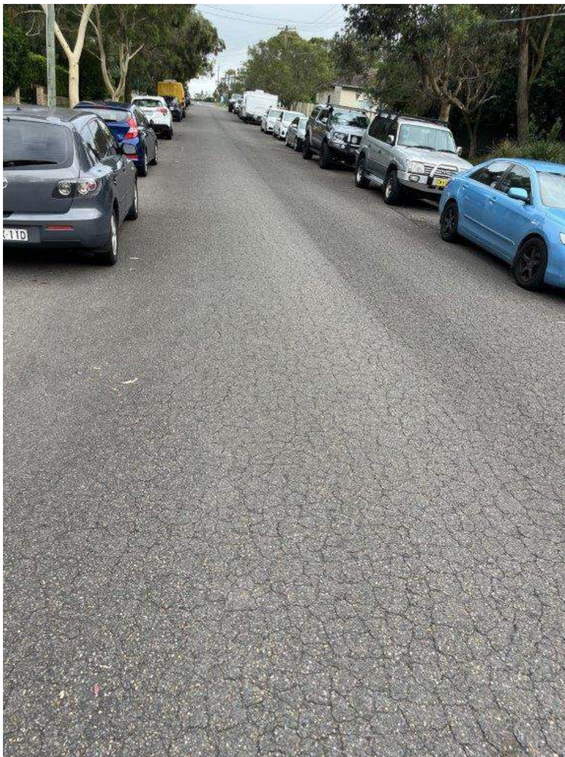
Photo 151 - Taren Point Road - Cracking of pavement
