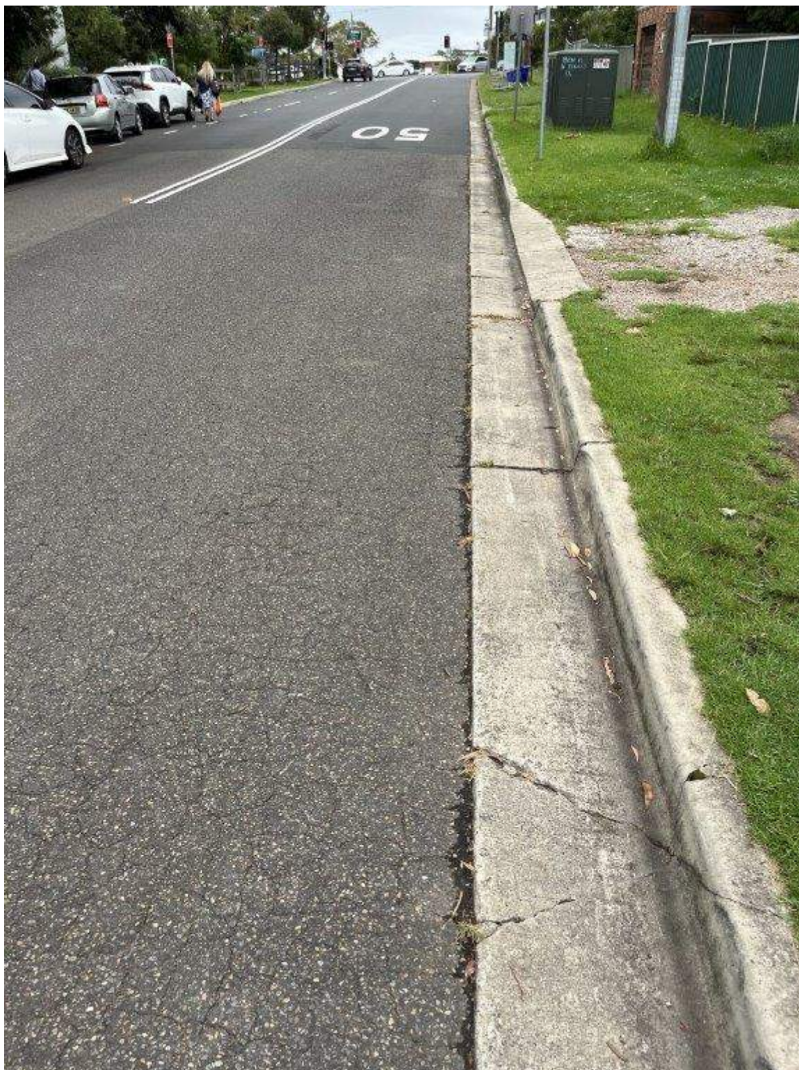
Photo 216 - Taren Point Road - Cracking of kerb and pavement
