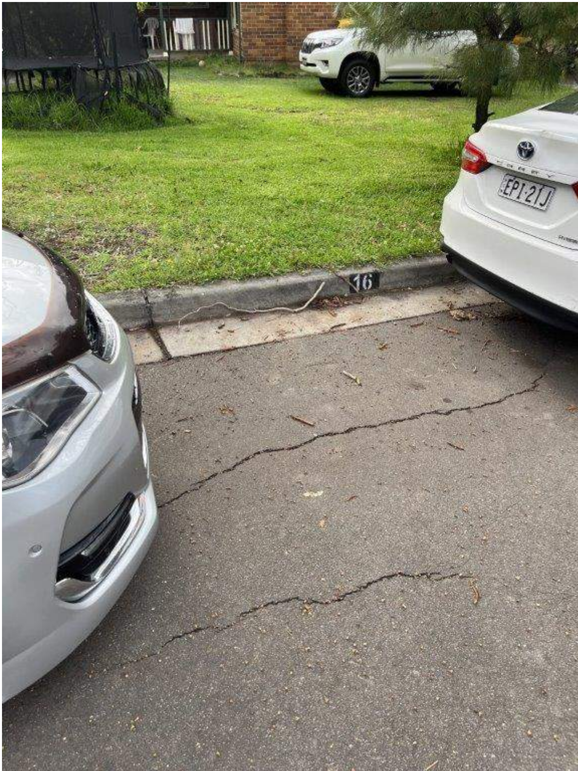
Photo 82 - Hinkler Avenue - Cracking of pavement
