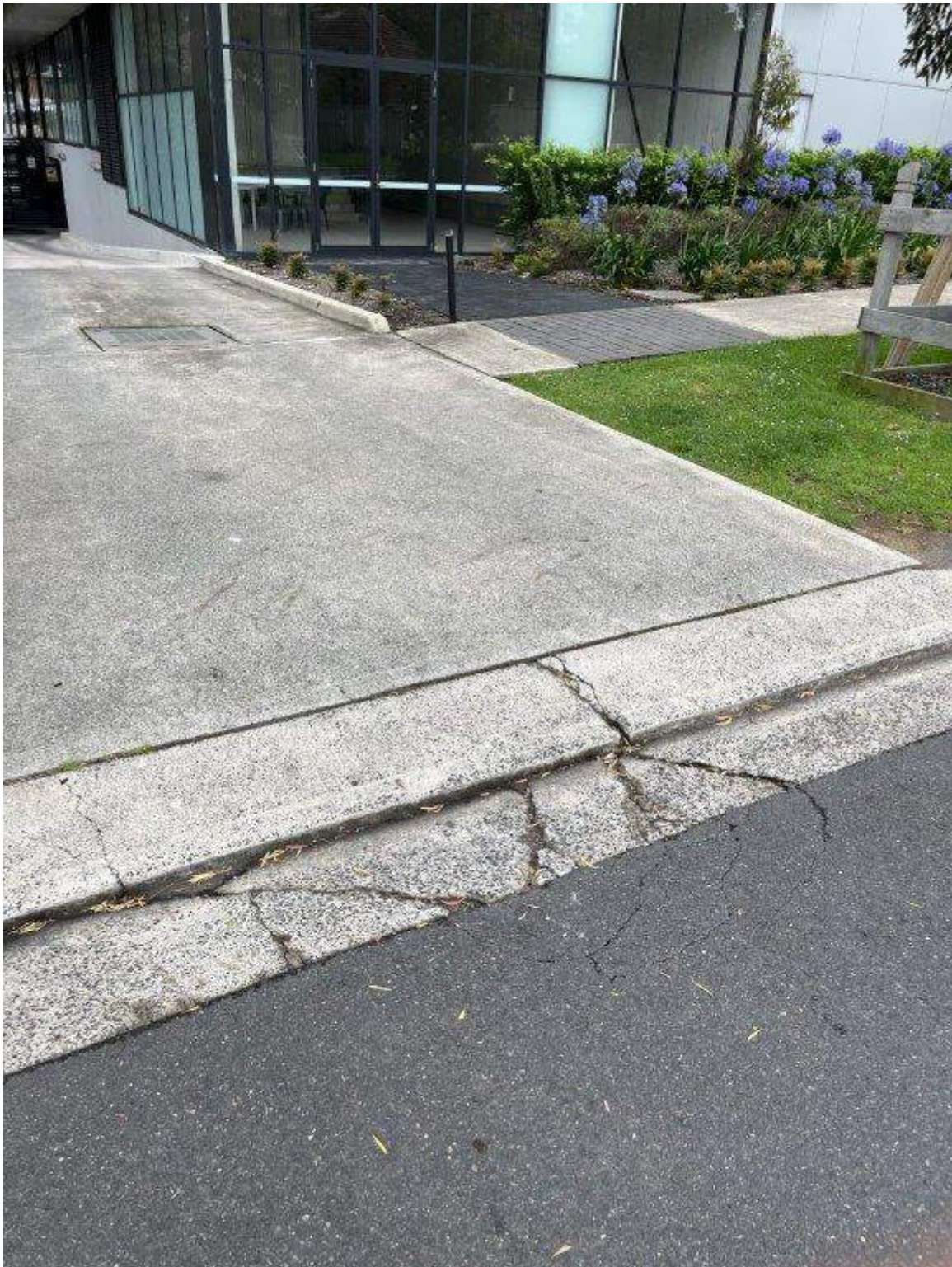
Photo 242 - Taren Point Road - Cracking of pavement
