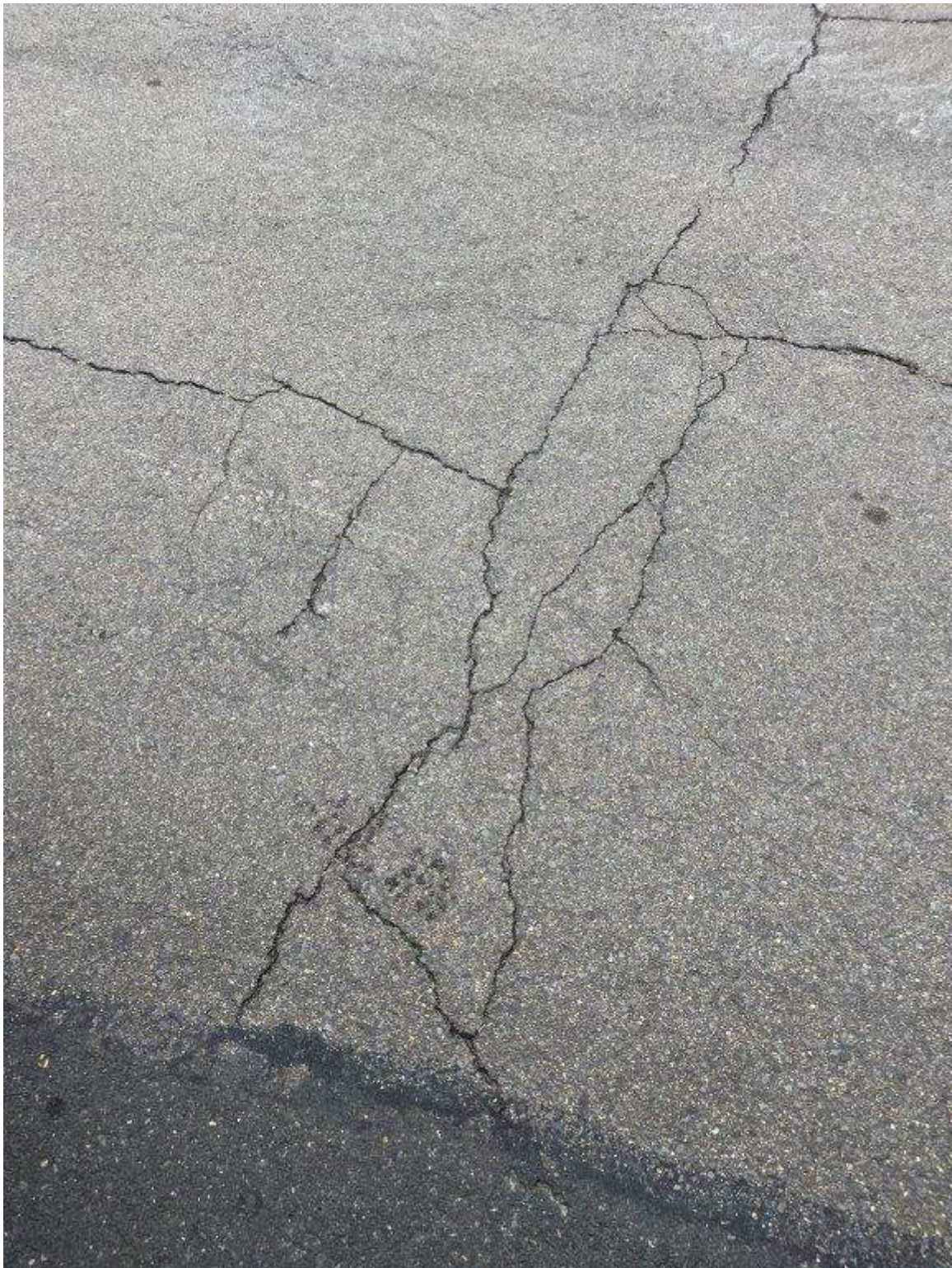
Photo 9 - Hinkler Avenue - Cracking of pavement
