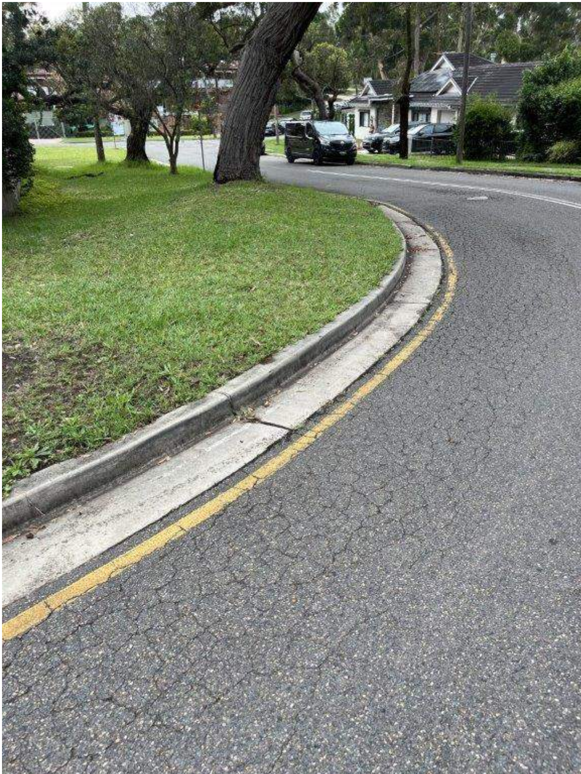
Photo 117 - Hinkler Avenue - Cracking of pavement
