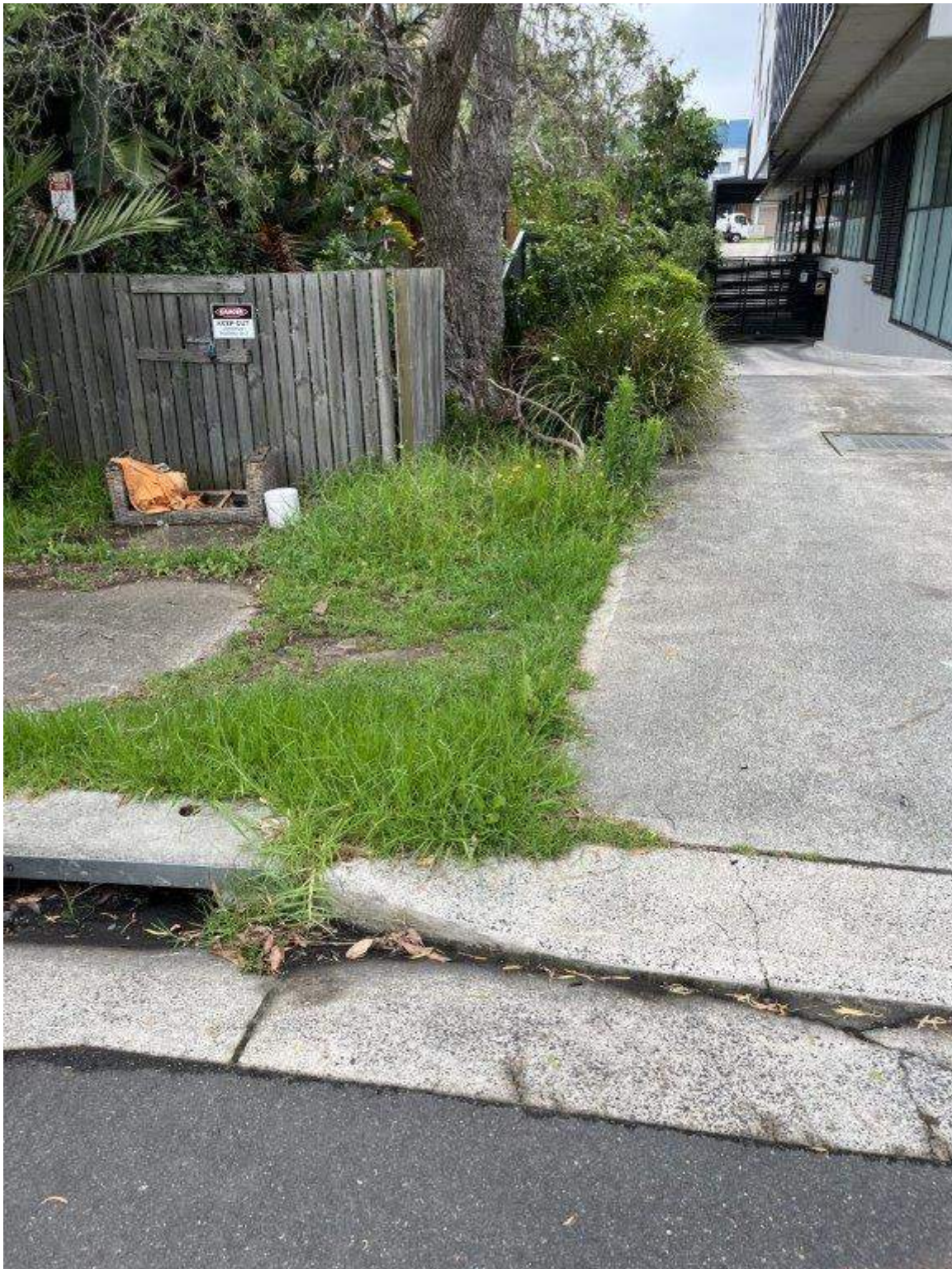
Photo 241 - Taren Point Road - Cracking of pavement
