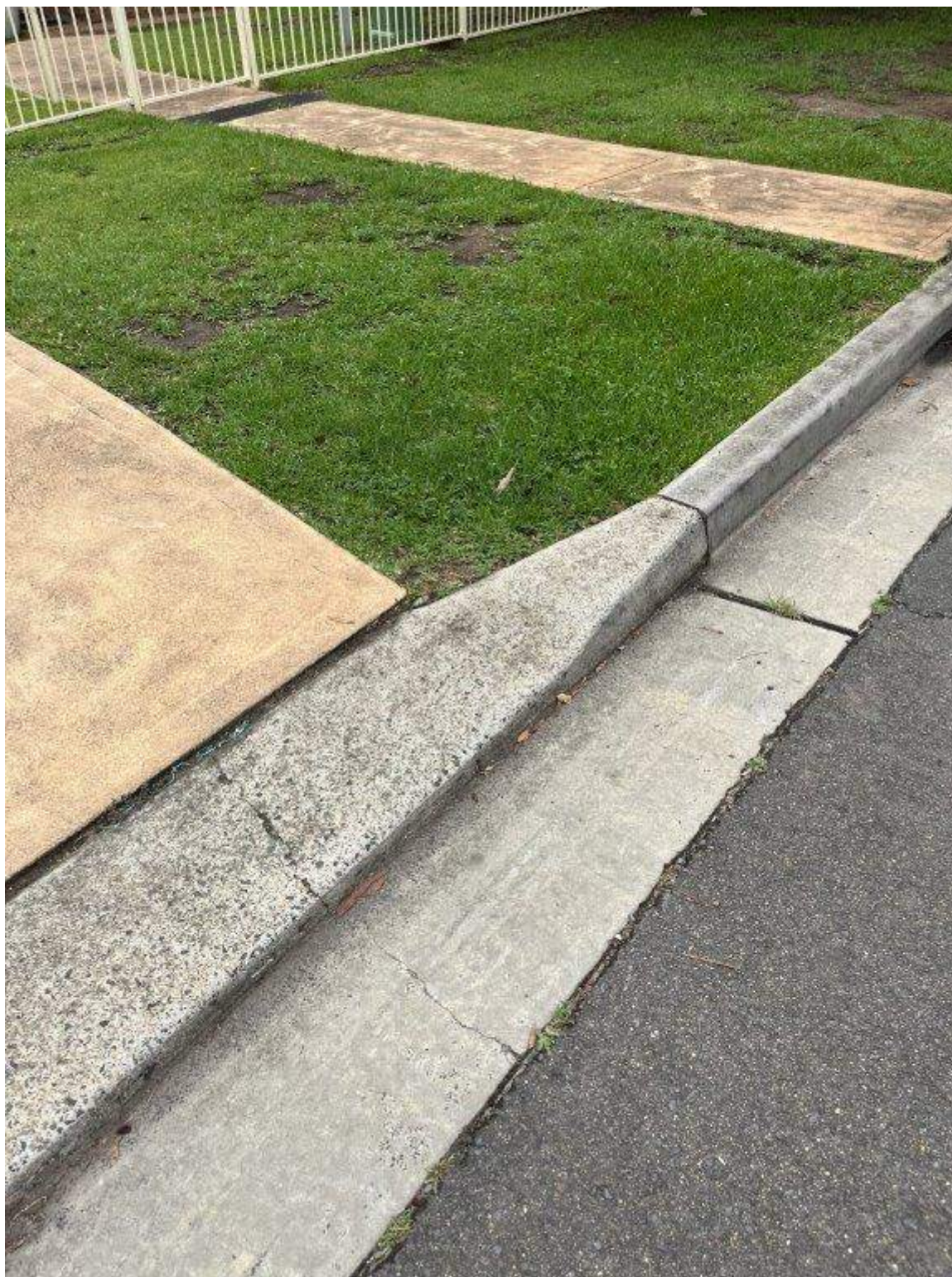
Photo 65 - Hinkler Avenue - Cracking of pavement
