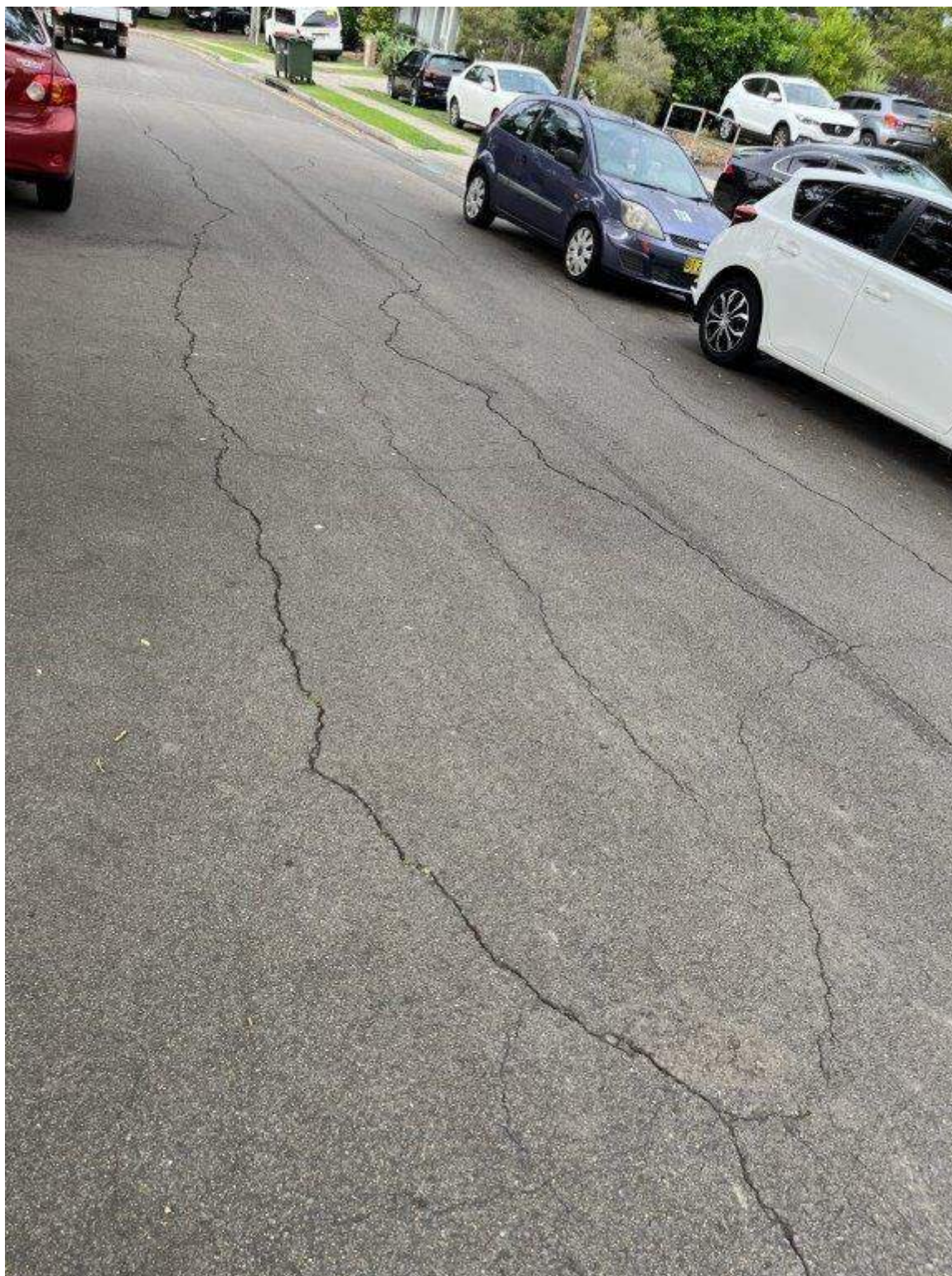
Photo 93 - Hinkler Avenue - Cracking of pavement
