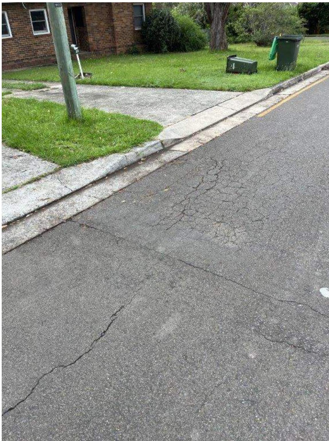
Photo 101 - Hinkler Avenue - Cracking of pavement
