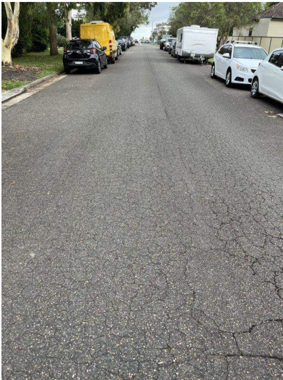
Photo 164 - Taren Point Road - Cracking of pavement
