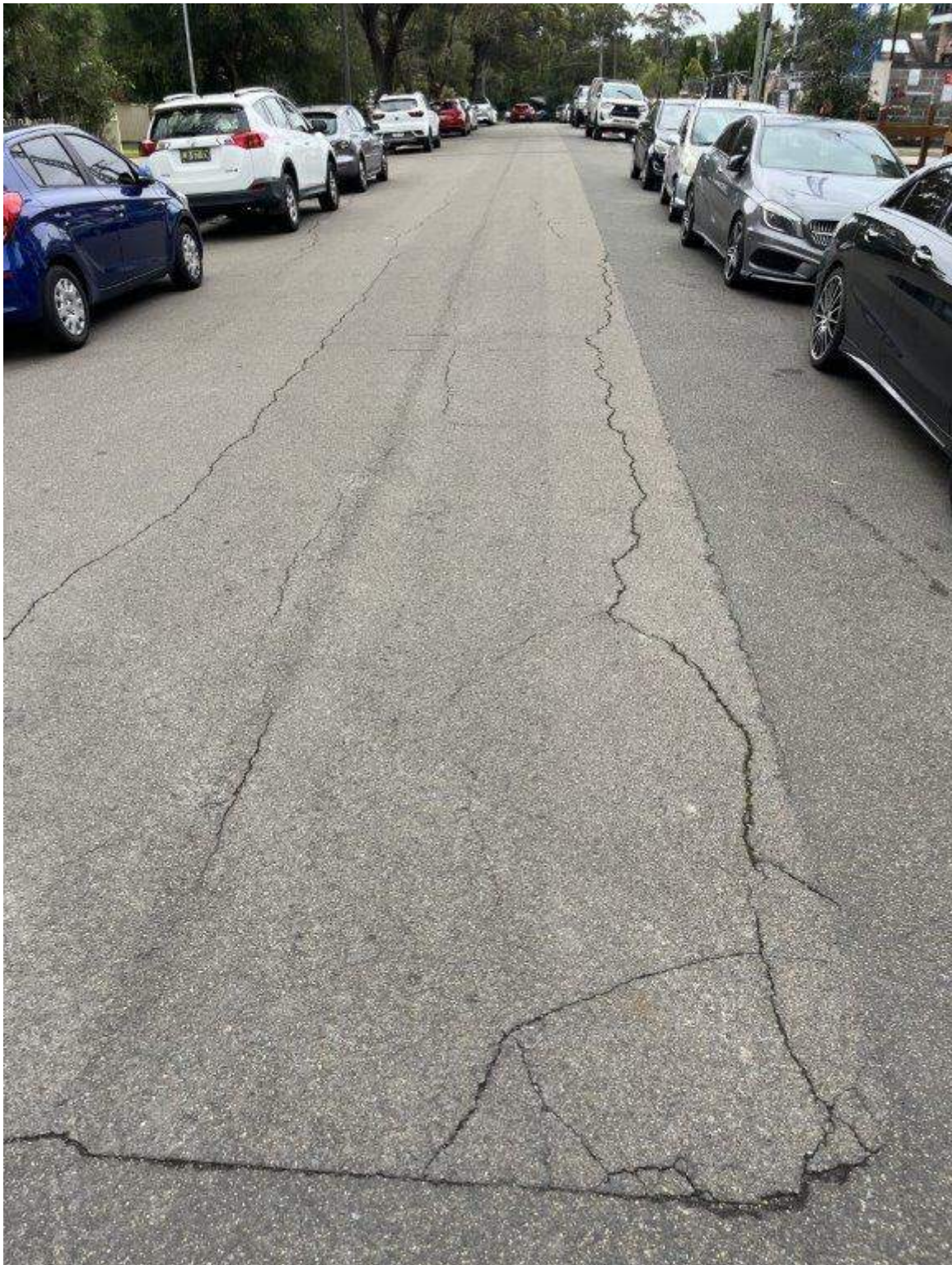
Photo 41 - Hinkler Avenue - Cracking of pavement
