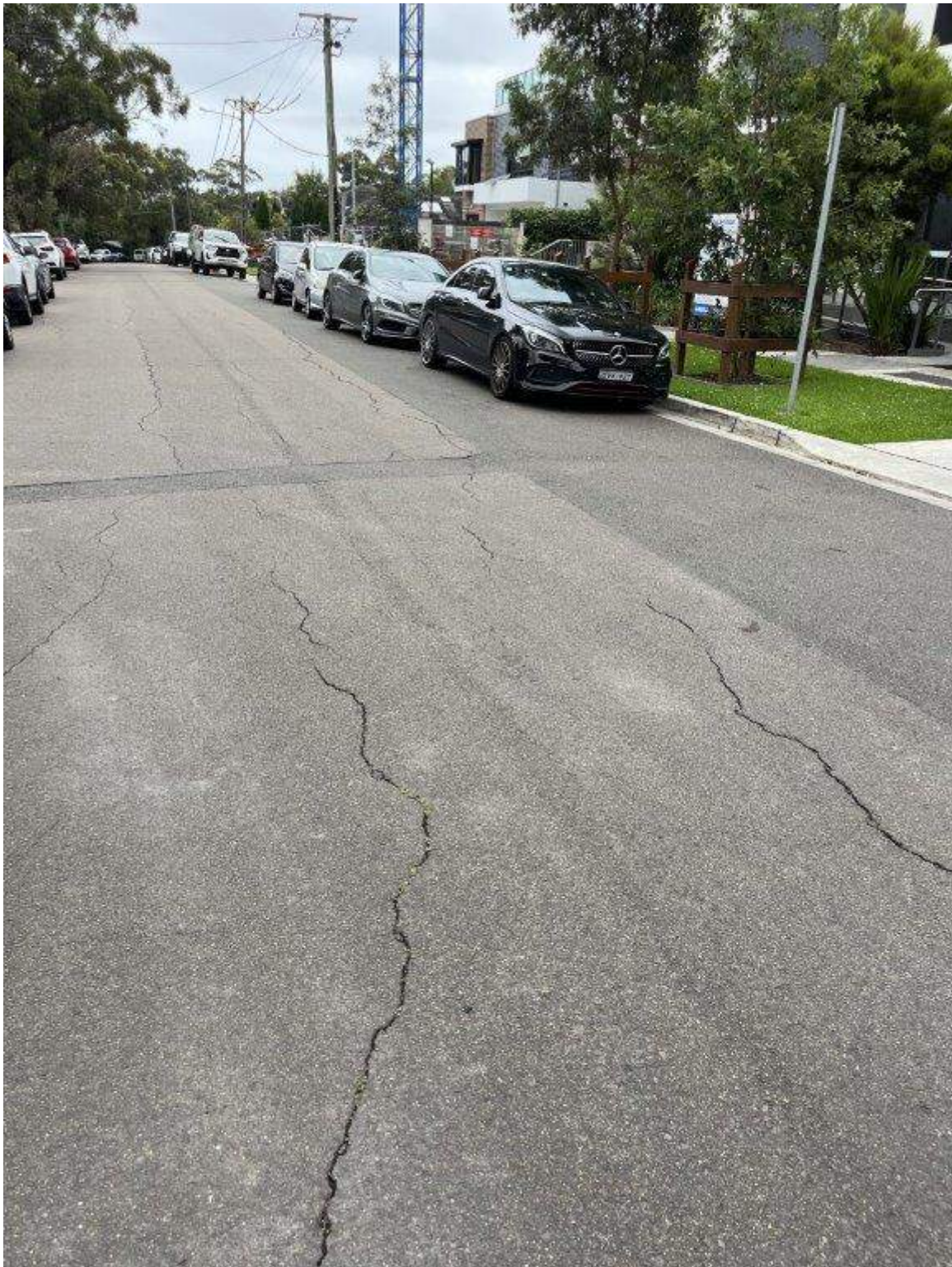
Photo 37 - Hinkler Avenue - Cracking of pavement
