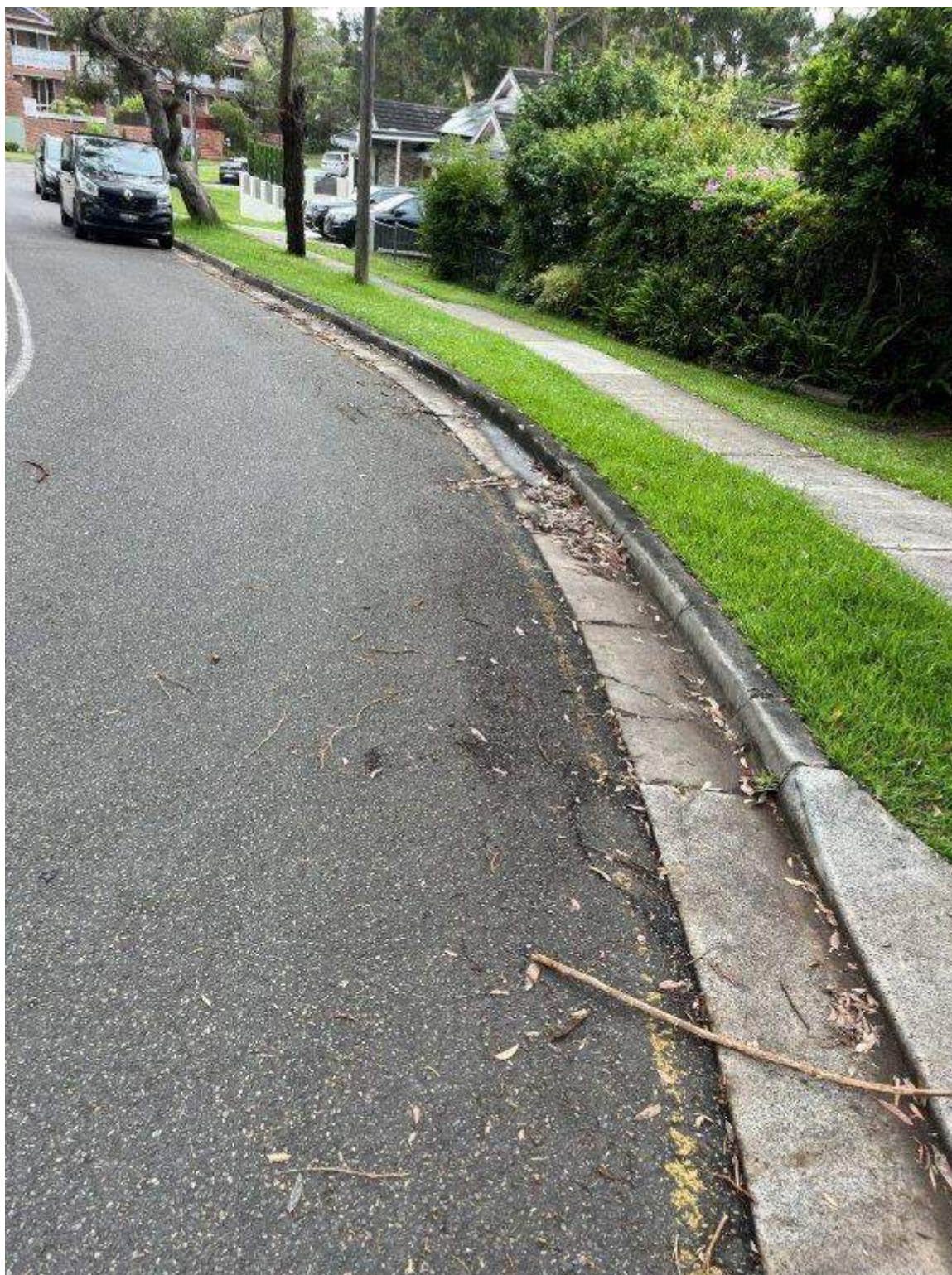
Photo 118 - Hinkler Avenue - Cracking of pavement
