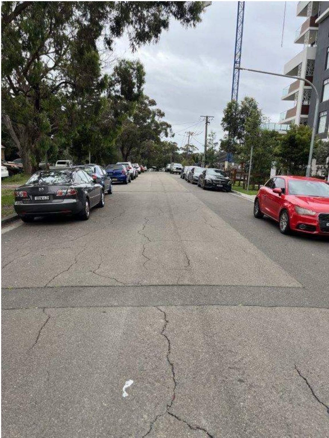
Photo 31 - Hinkler Avenue - Cracking of pavement
