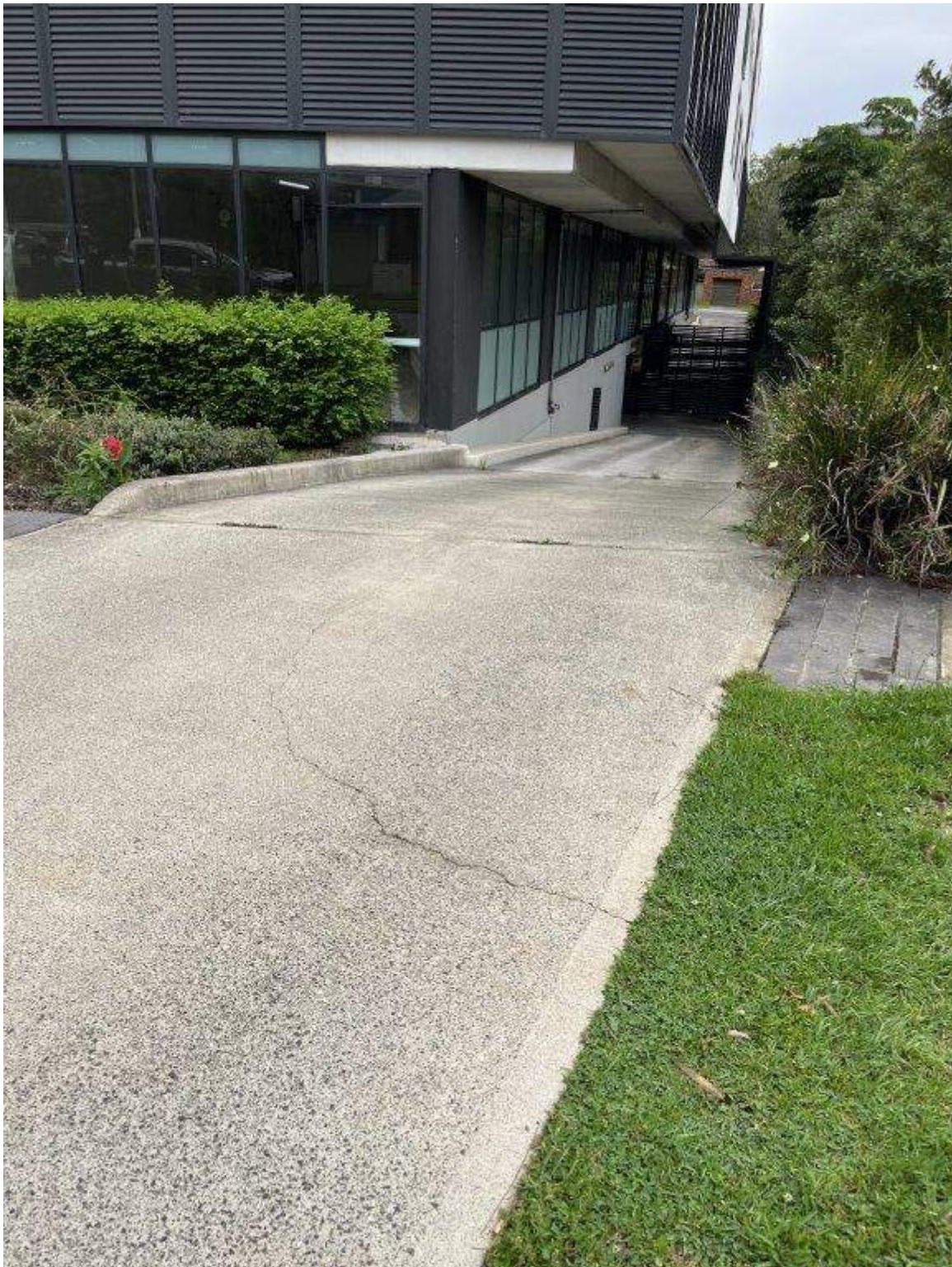
Photo 22 - Hinkler Avenue - Cracking of pavement
