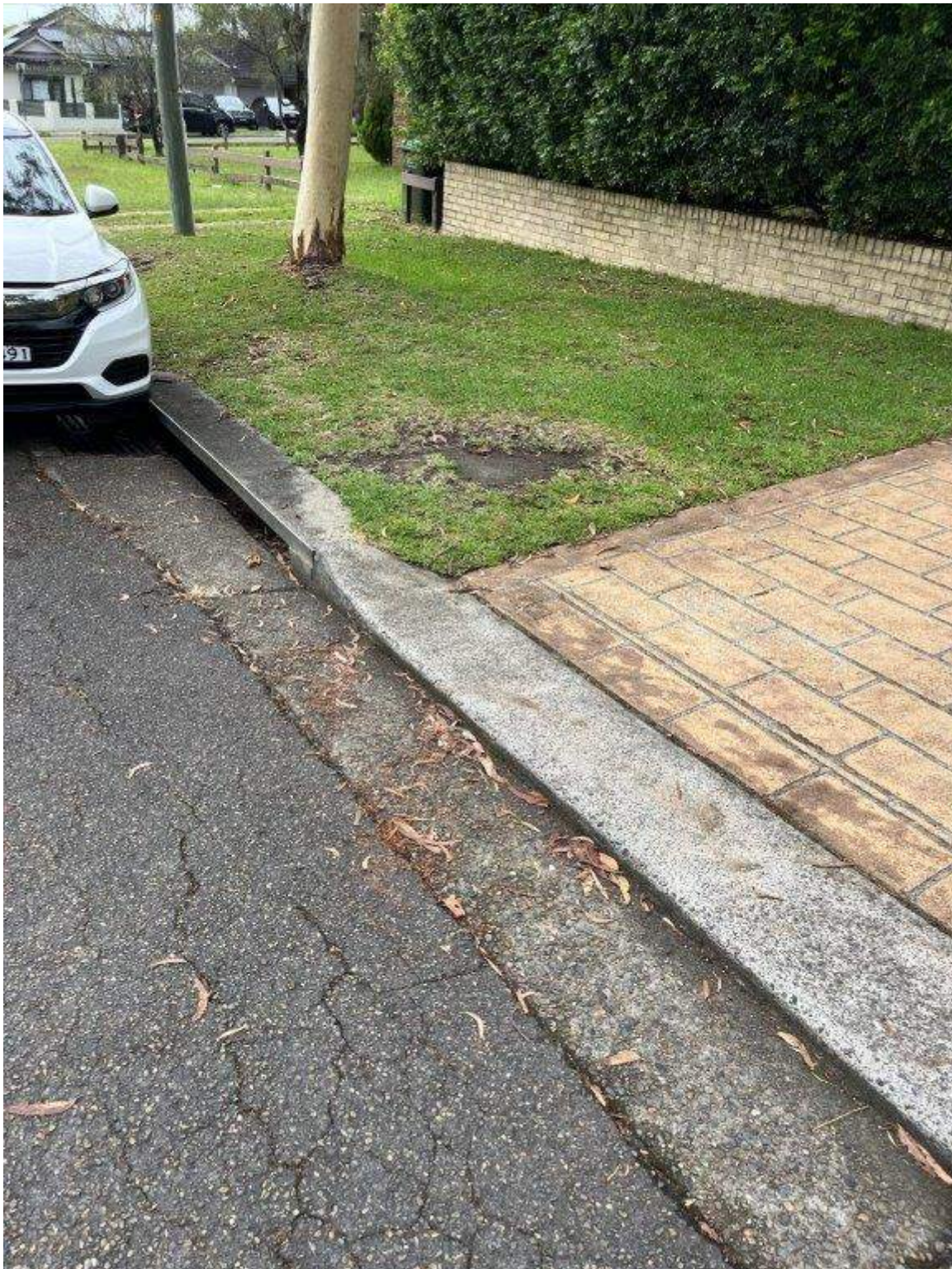
Photo 166 - Taren Point Road - Cracking of pavement
