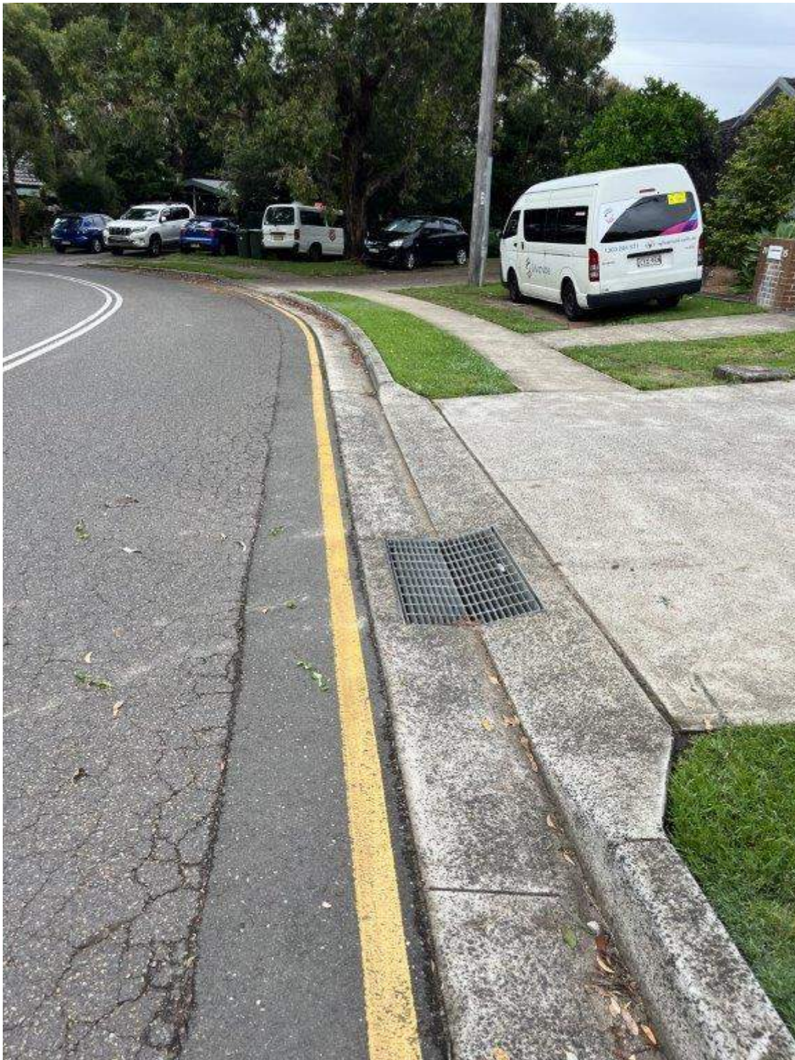
Photo 106 - Hinkler Avenue - Cracking of pavement
