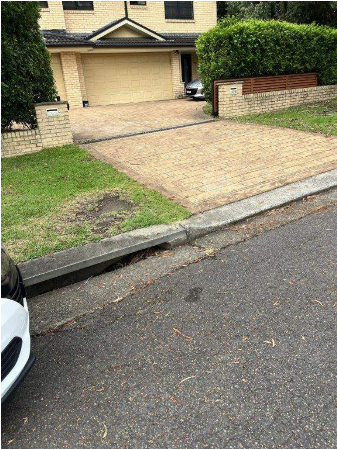
Photo 165 - Taren Point Road - Cracking of pavement
