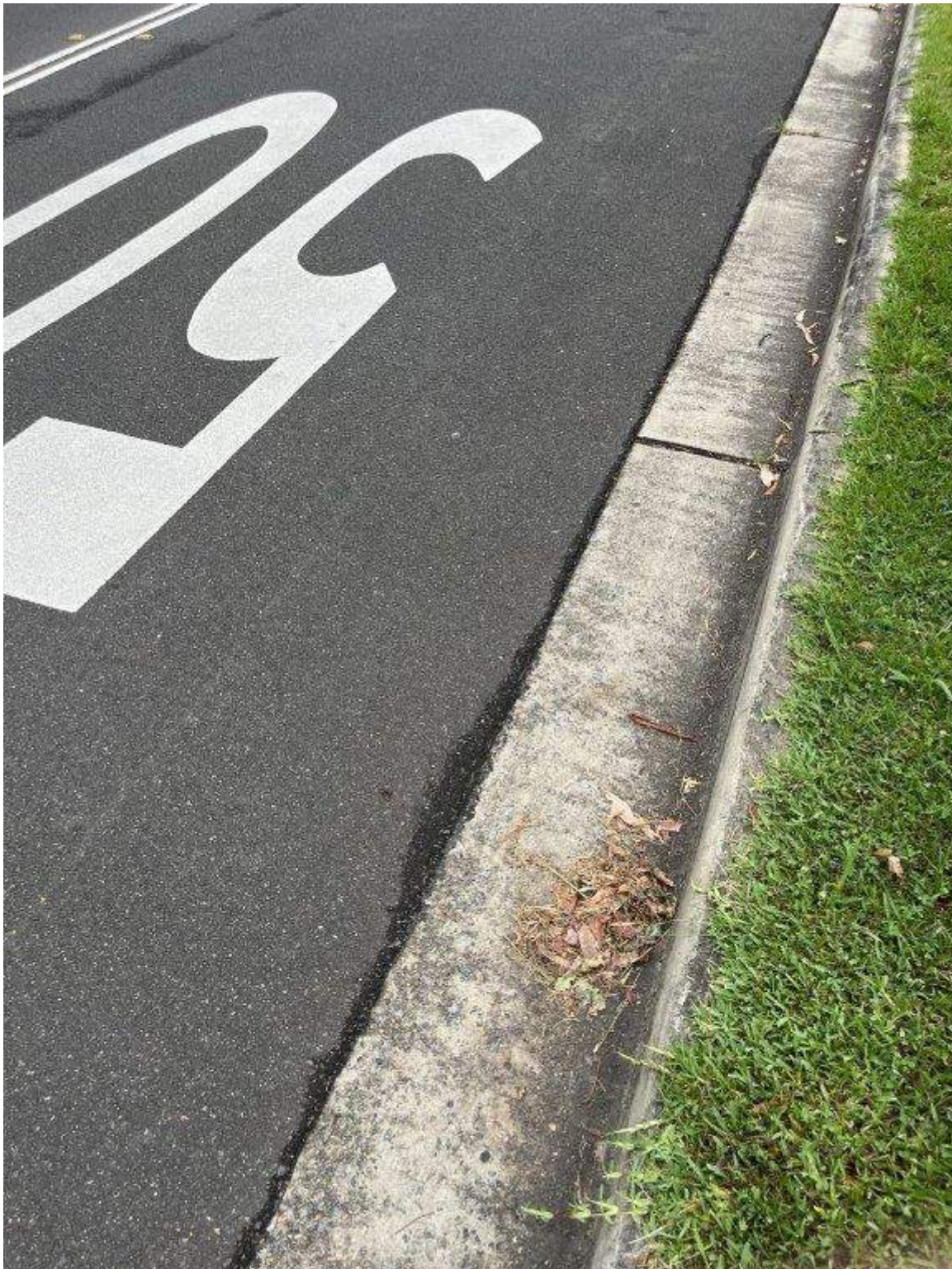
Photo 225 - Taren Point Road - Existing condition of pavement
