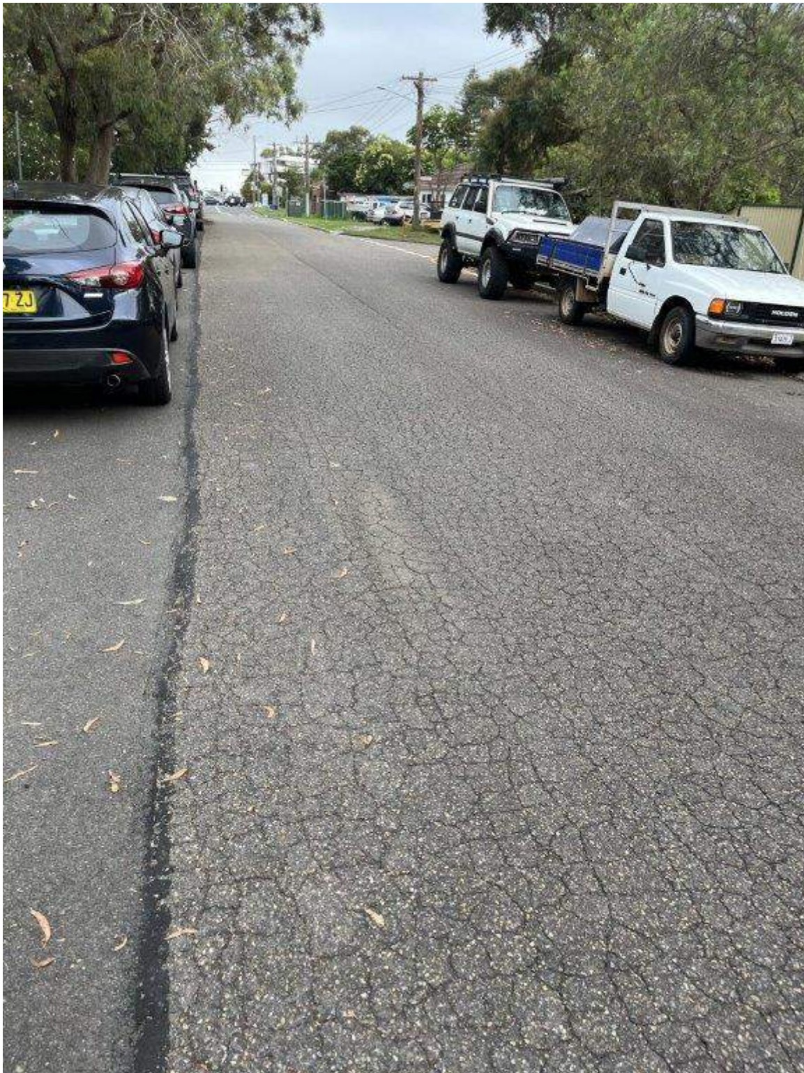
Photo 177 - Taren Point Road - Cracking of pavement
