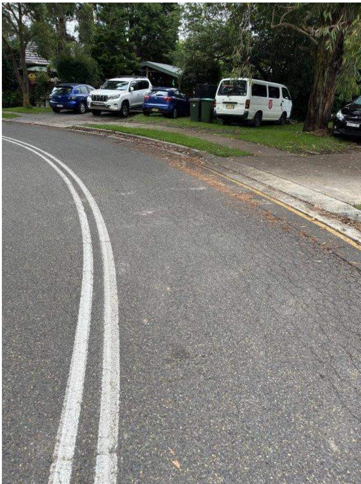
Photo 109 - Hinkler Avenue - Cracking of pavement
