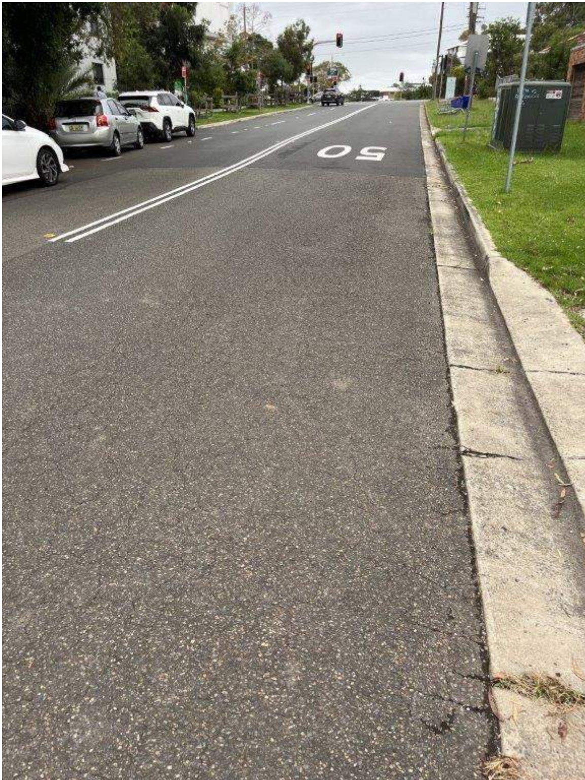
Photo 218 - Taren Point Road - Cracking of pavement
