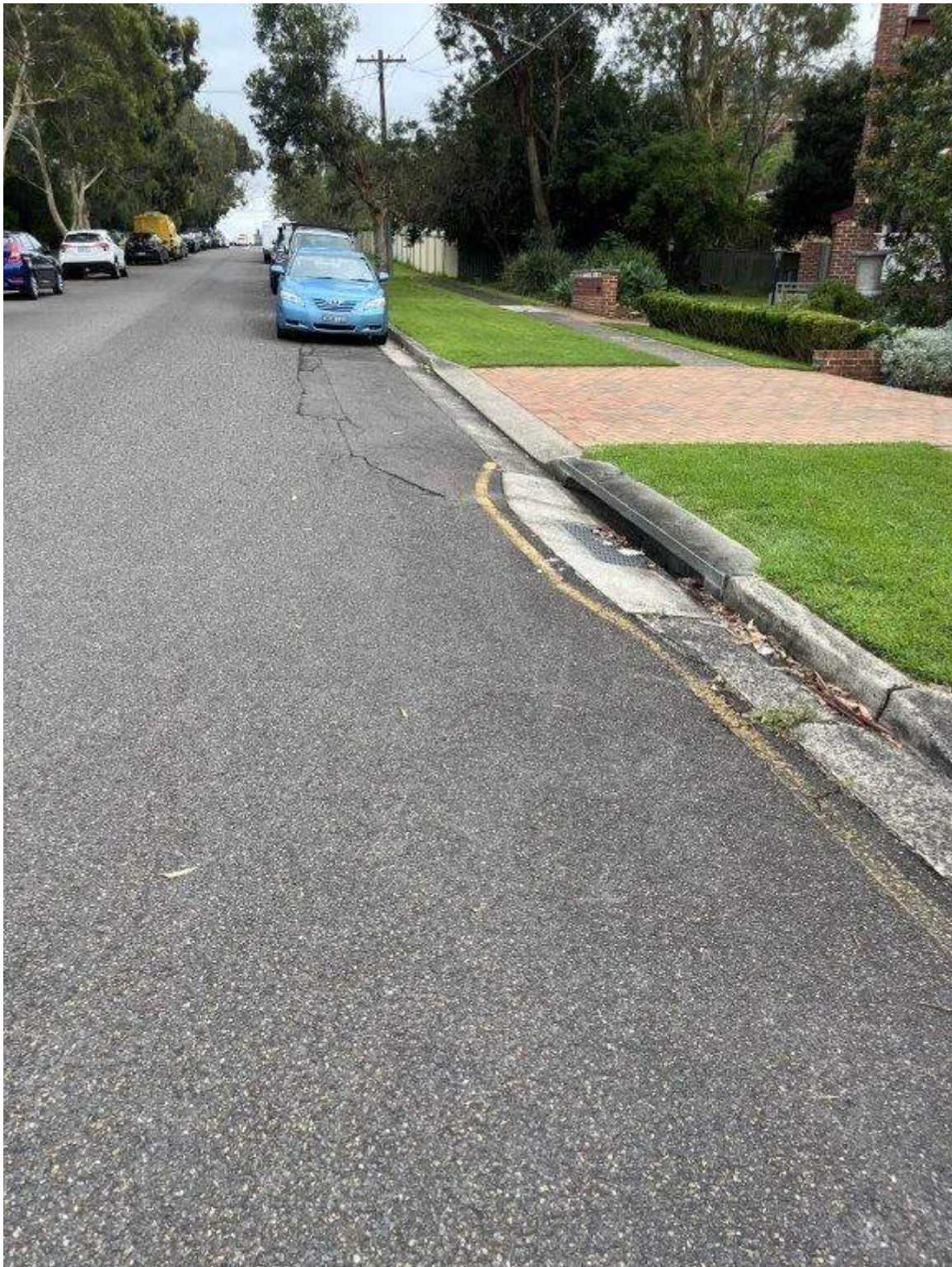
Photo 144 - Taren Point Road - Cracking of pavement
