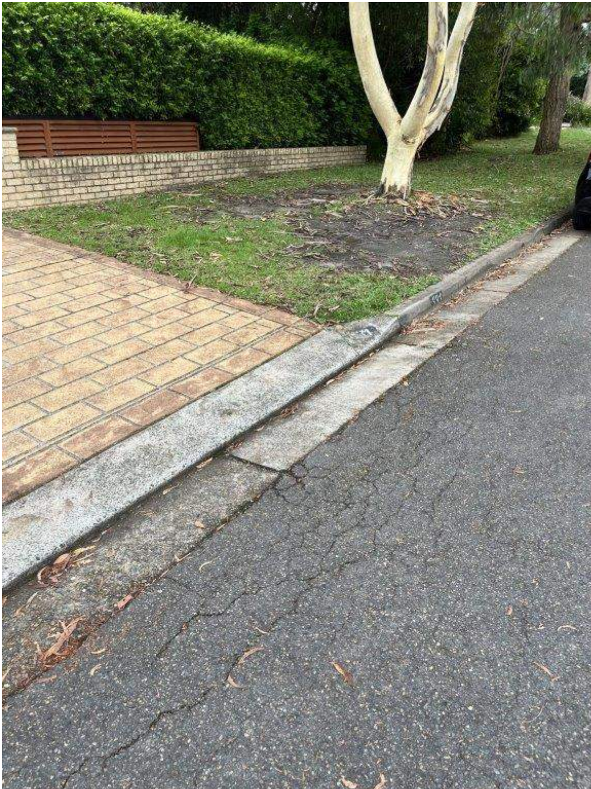
Photo 167 - Taren Point Road - Cracking of pavement
