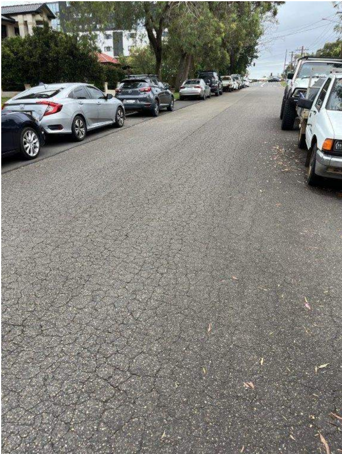
Photo 181 - Taren Point Road - Cracking of pavement
