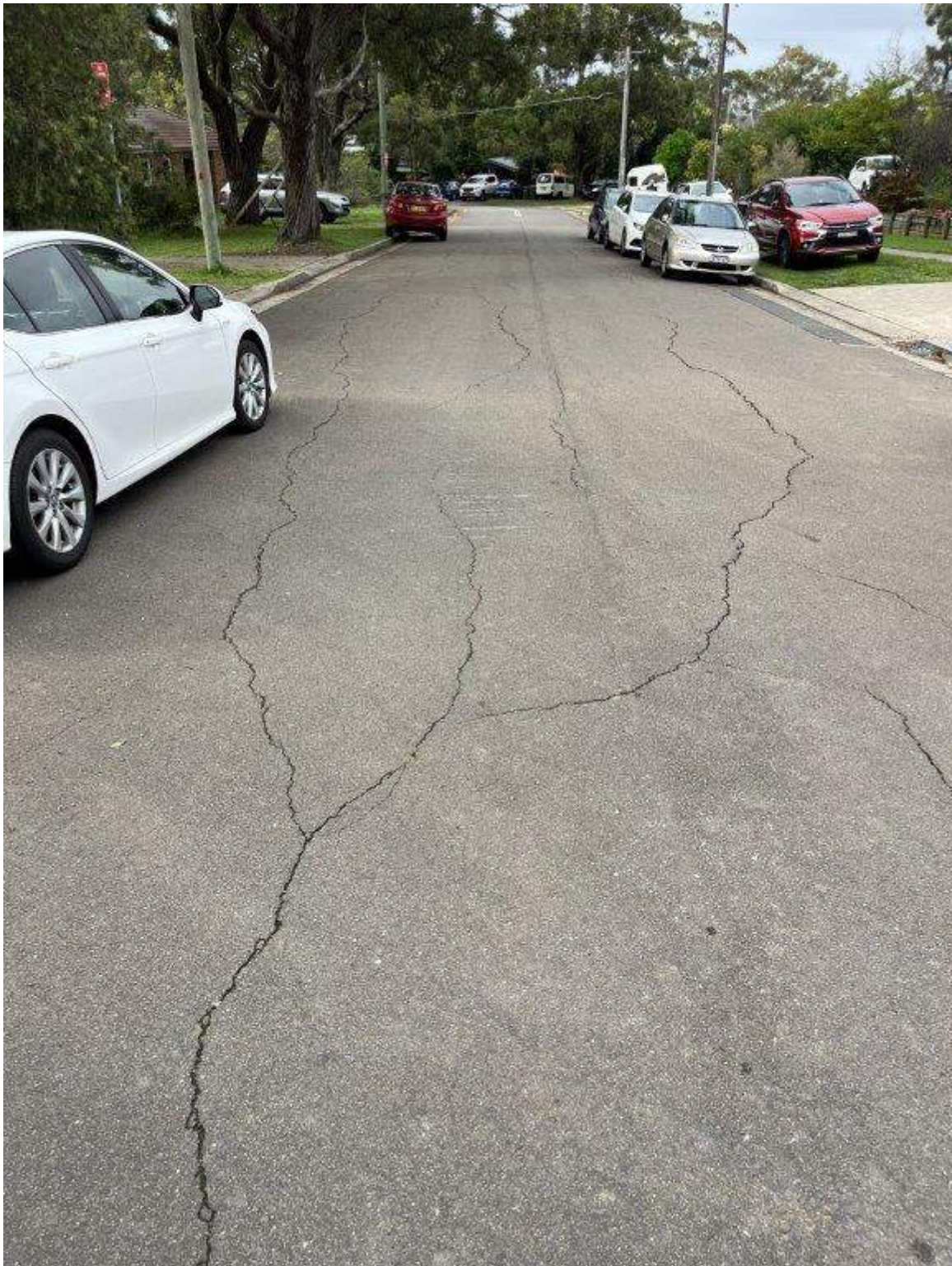
Photo 81 - Hinkler Avenue - Cracking of pavement
