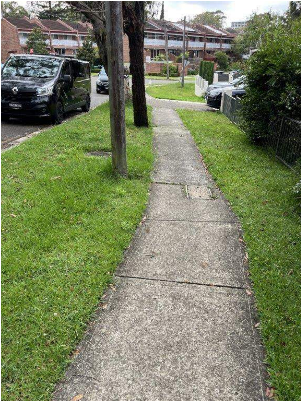
Photo 127 - Hinkler Avenue - Differential settlement of pavement
