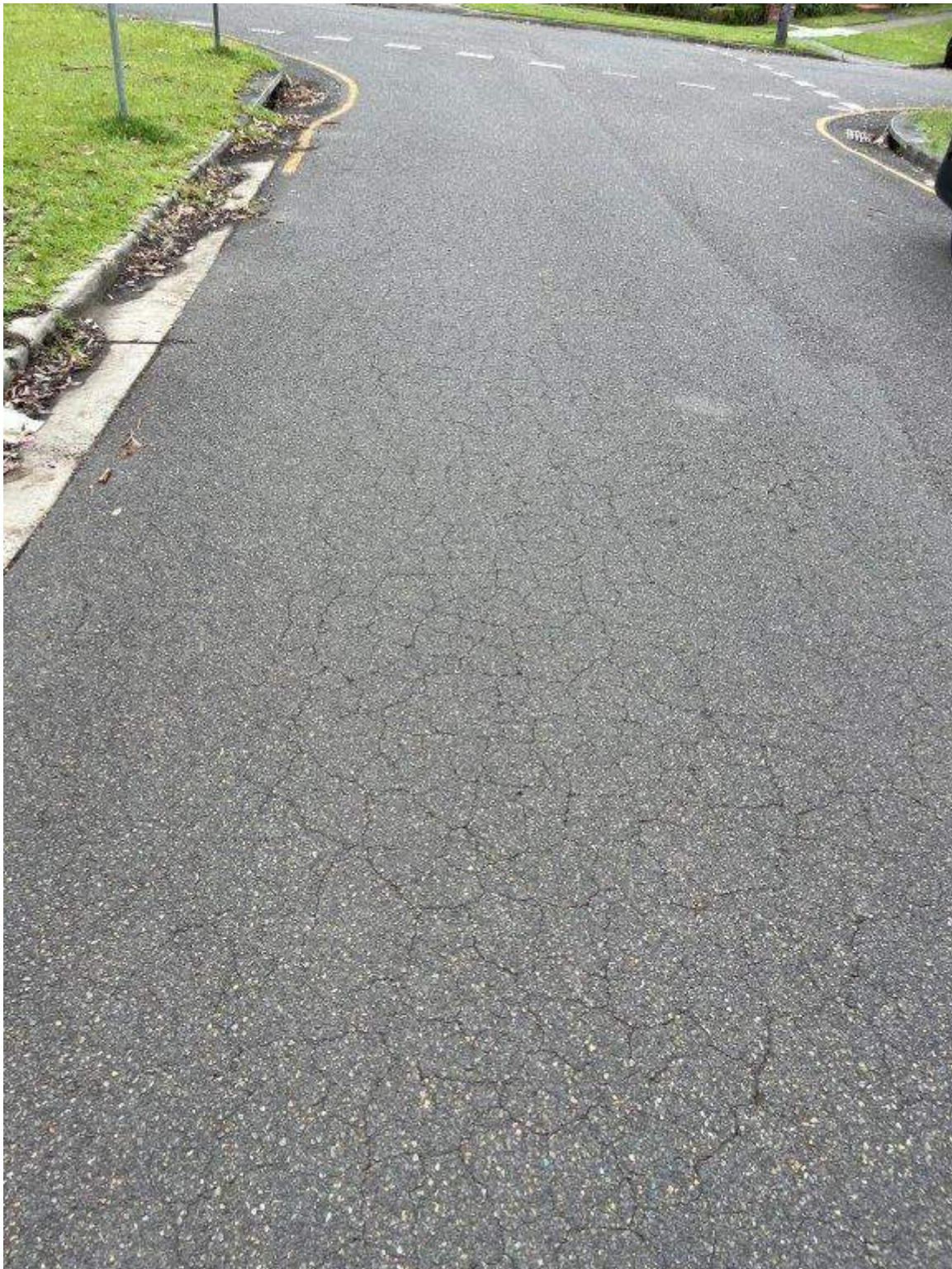
Photo 136 - Hinkler Avenue - Cracking of pavement
