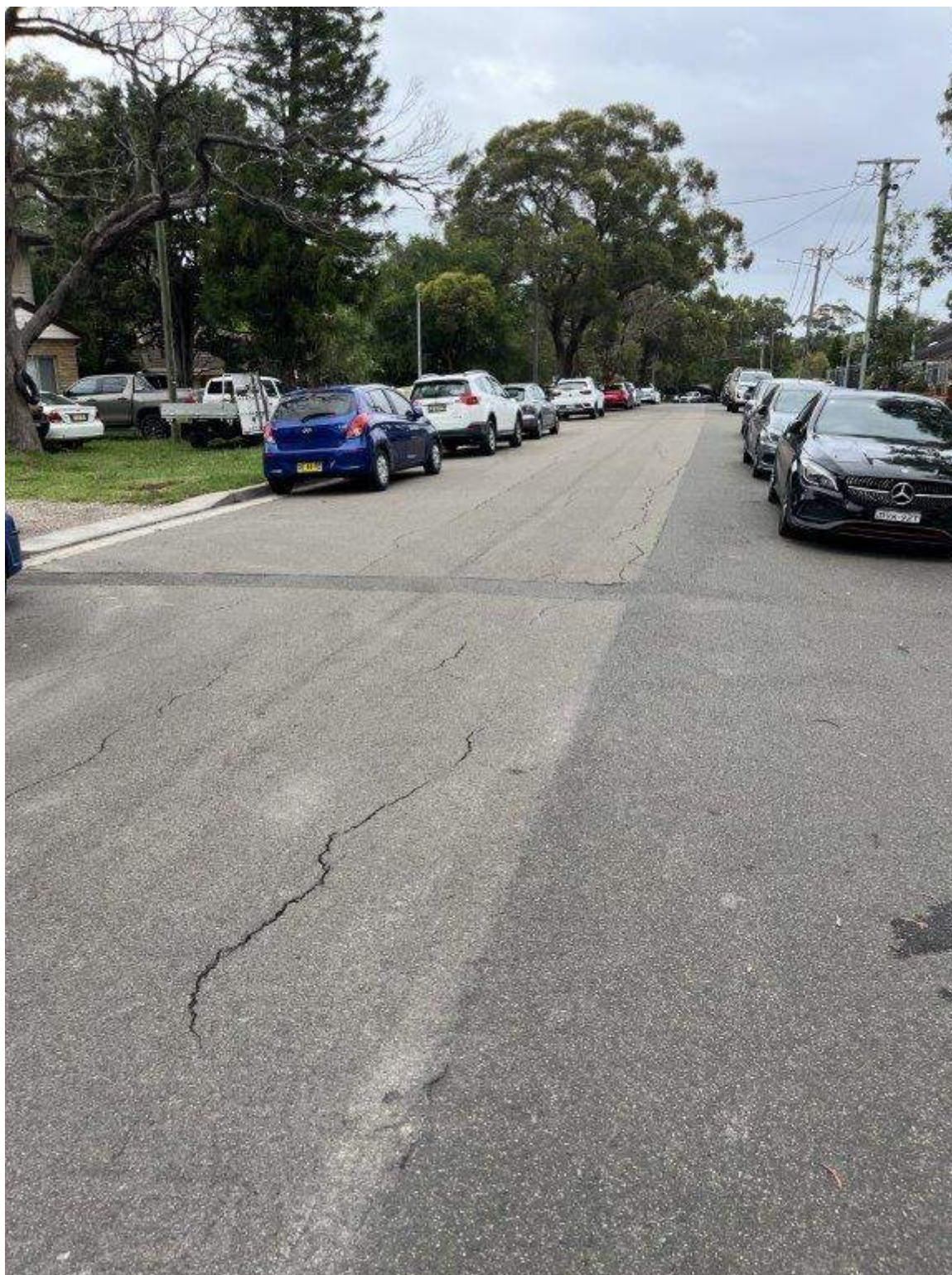
Photo 50 - Hinkler Avenue - Cracking of pavement
