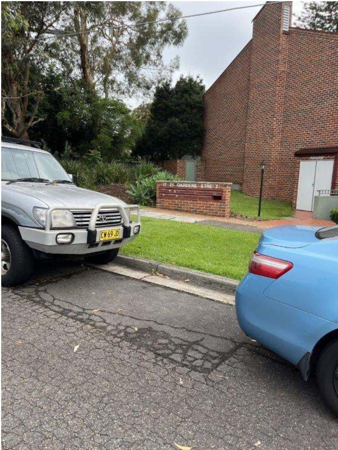
Photo 153 - Taren Point Road - Cracking of pavement
