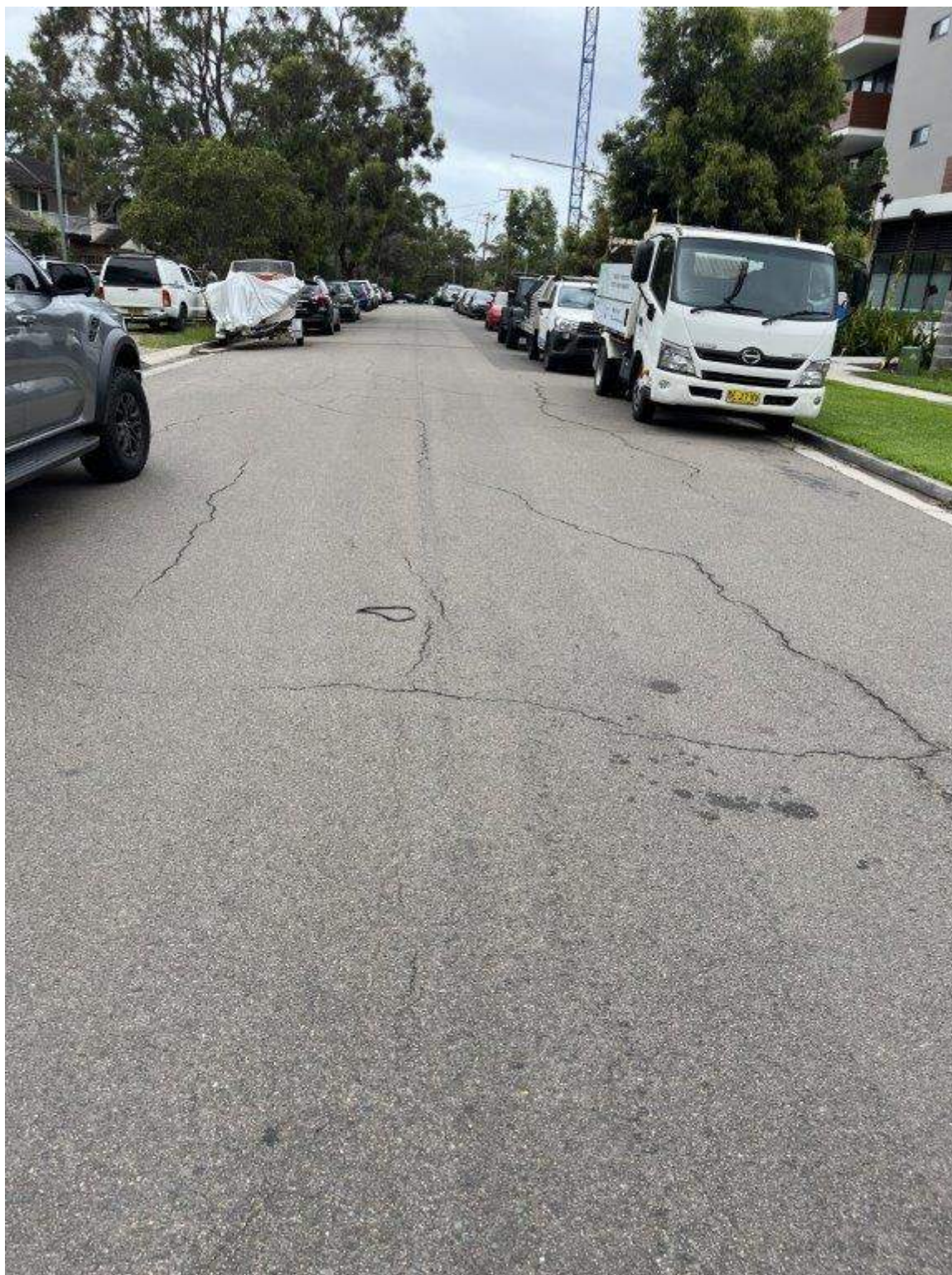
Photo 16 - Hinkler Avenue - Cracking of pavement
