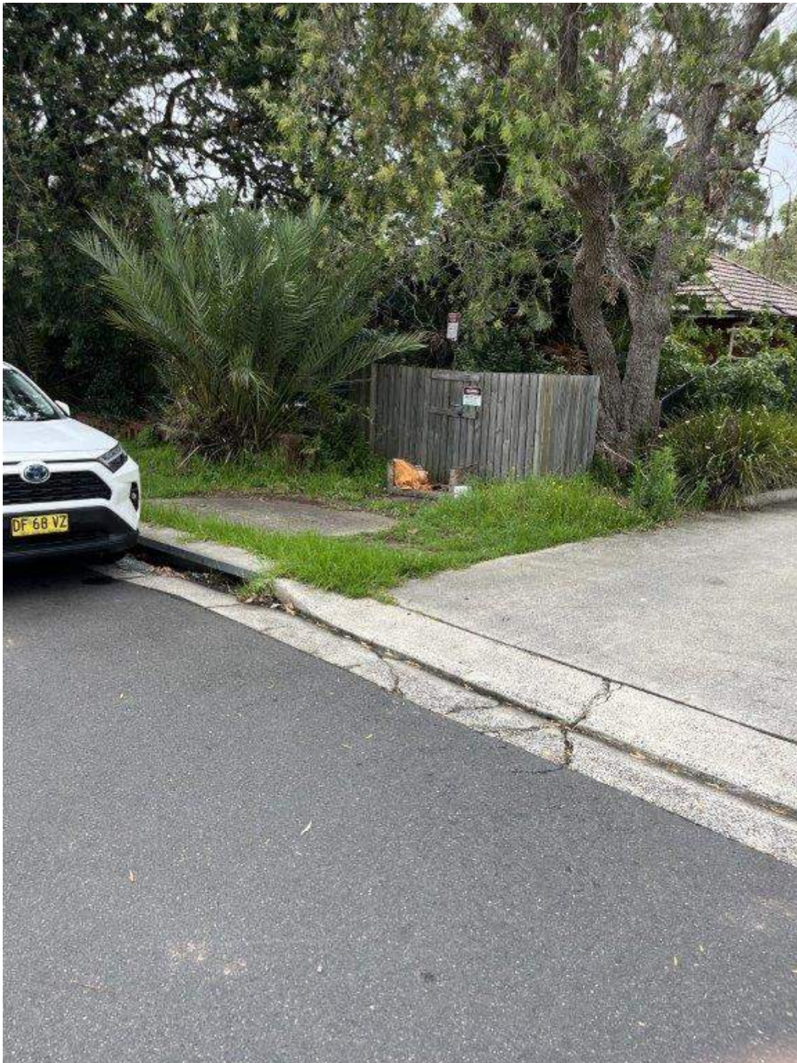
Photo 239 - Taren Point Road - Cracking of pavement
