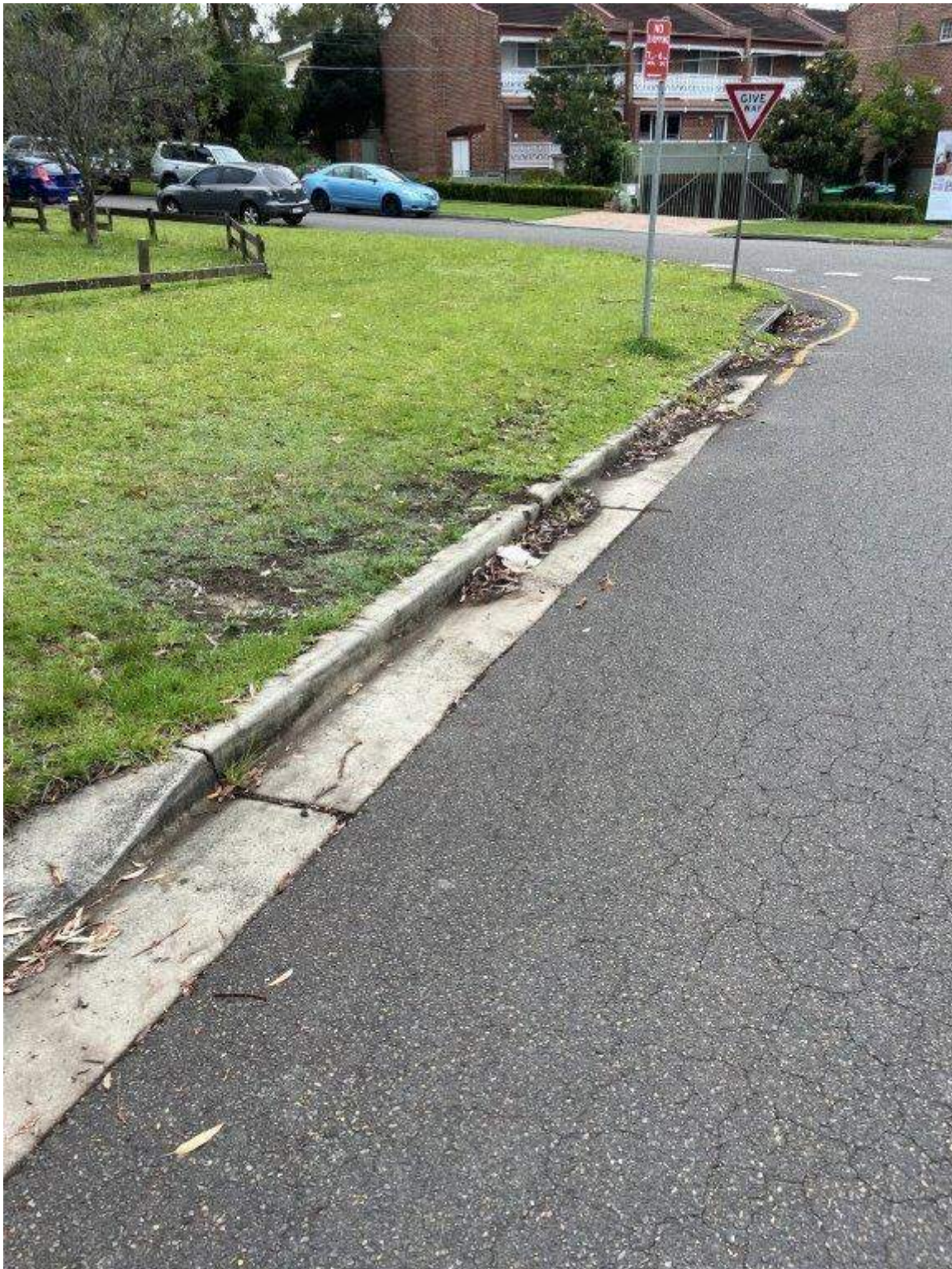
Photo 135 - Hinkler Avenue - Cracking of pavement
