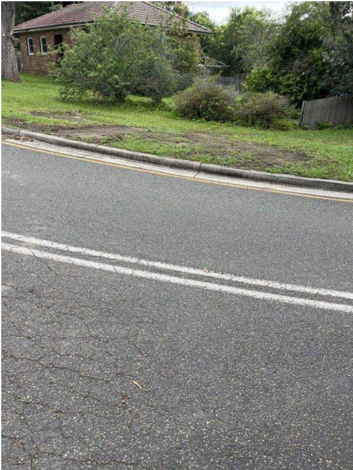
Photo 113 - Hinkler Avenue - Cracking of pavement
