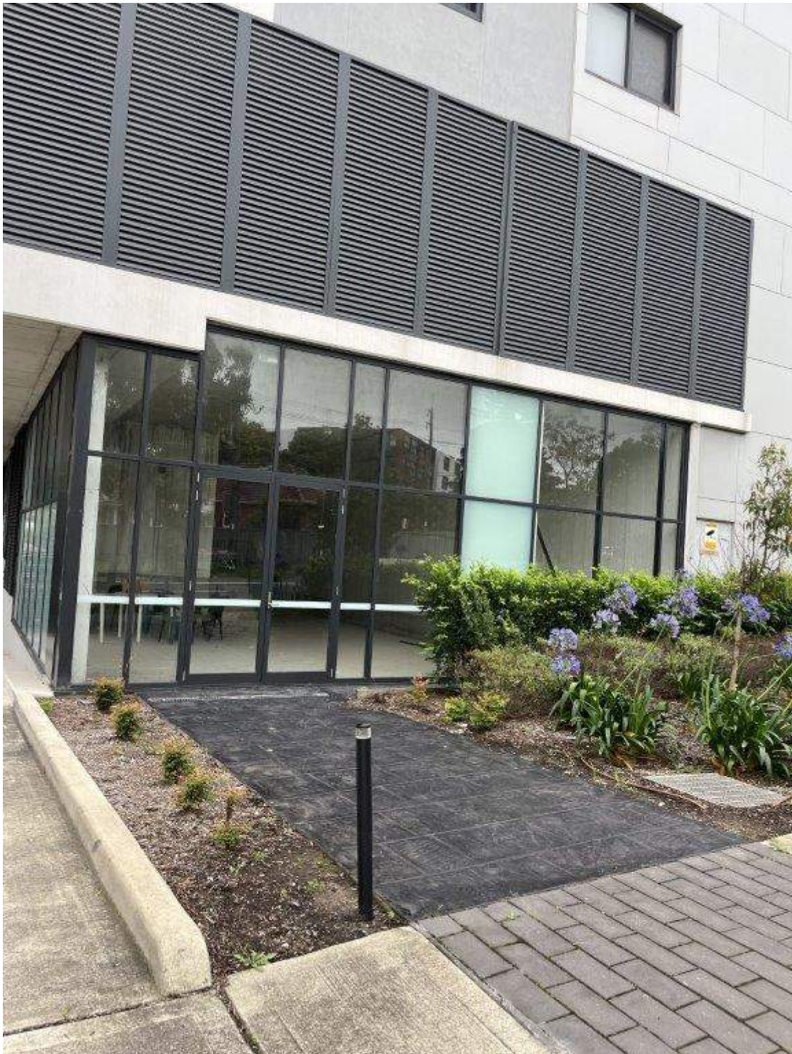
Photo 245 - Taren Point Road - Existing condition of external façade and pavement
