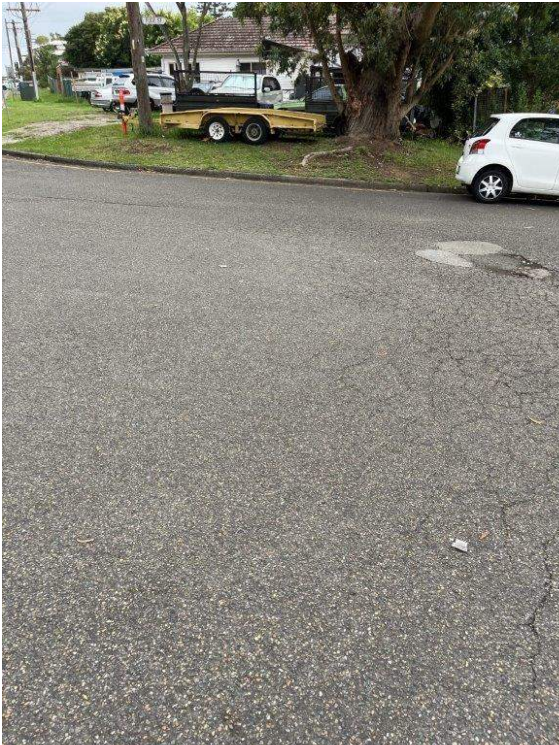
Photo 187 - Taren Point Road - Cracking of pavement
