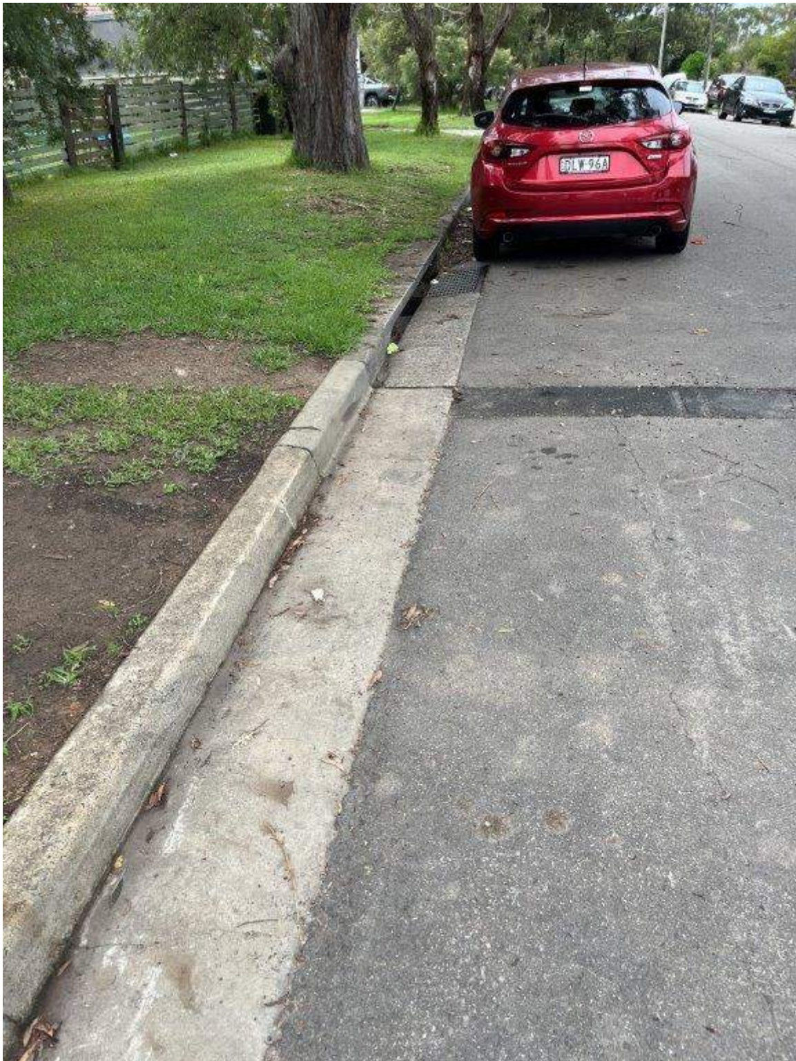
Photo 71 - Hinkler Avenue - Cracking of pavement
