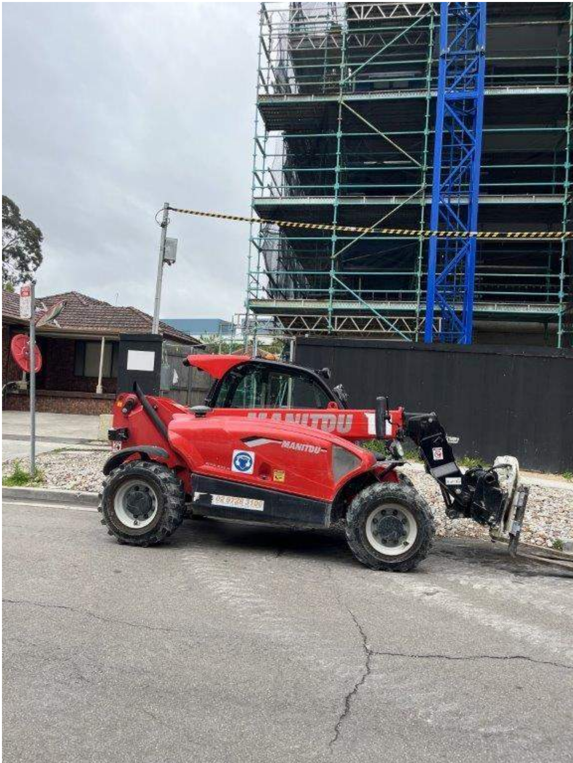
Photo 8 - Hinkler Avenue - Cracking of pavement
