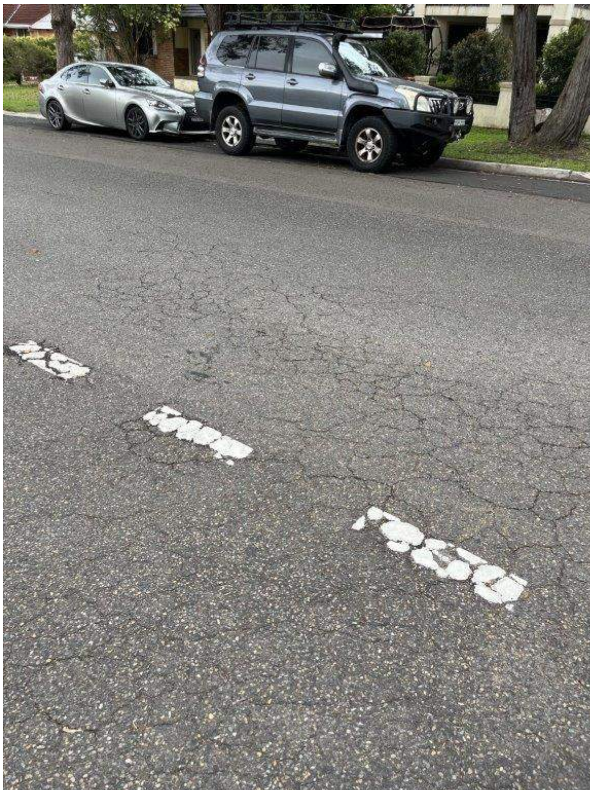
Photo 203 - Taren Point Road - Cracking of pavement
