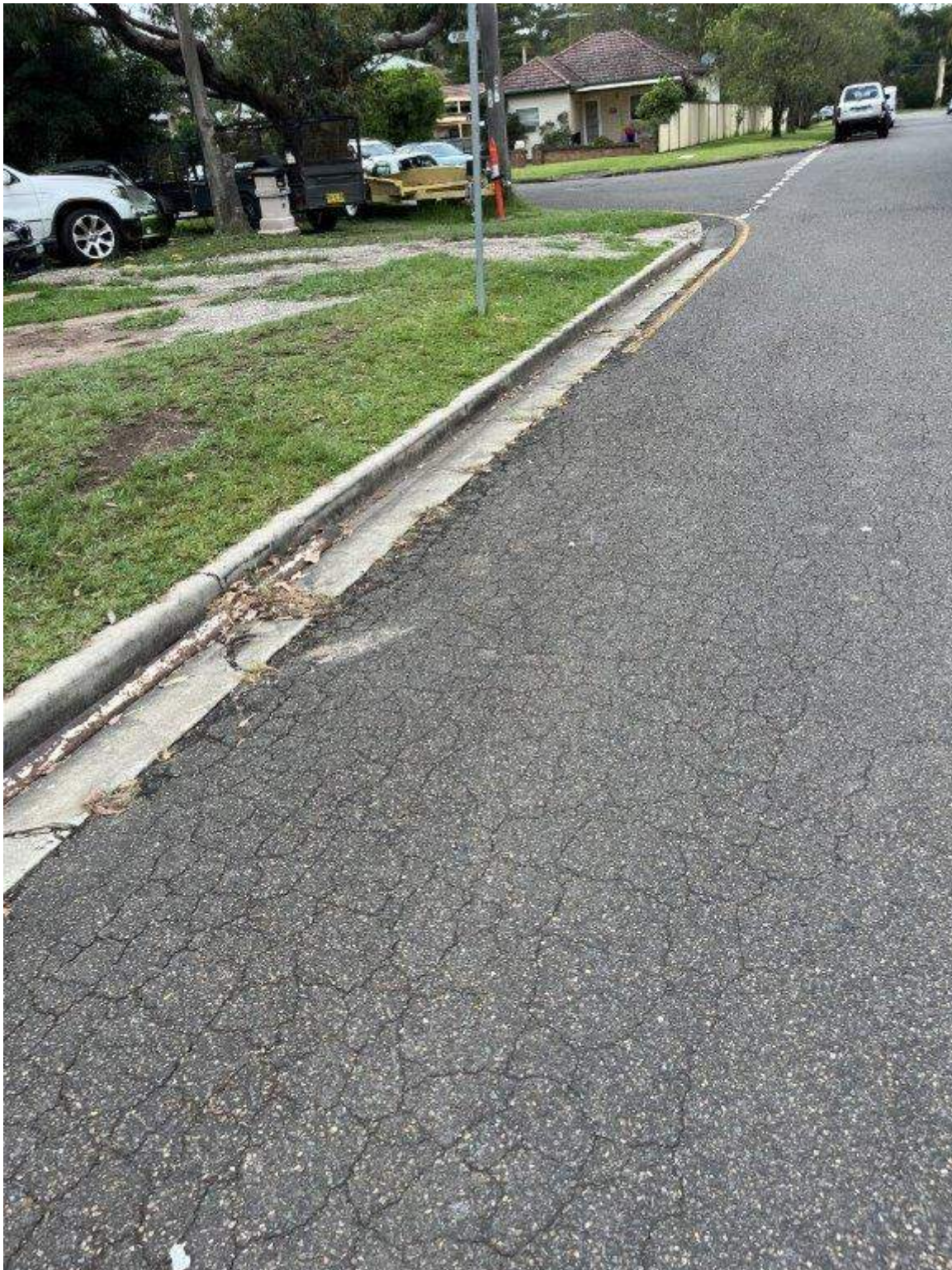
Photo 213 - Taren Point Road - Cracking of pavement
