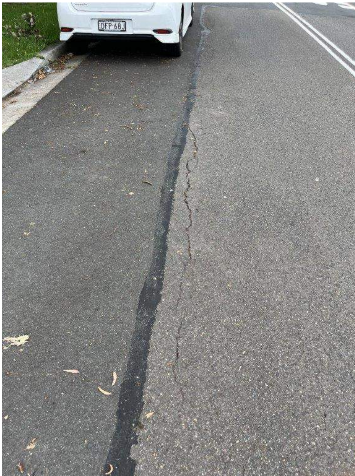
Photo 220 - Taren Point Road - Cracking of pavement
