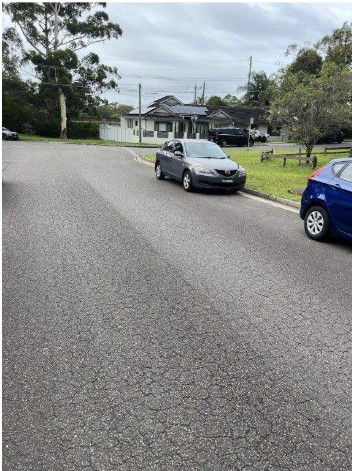
Photo 158 - Taren Point Road - Cracking of pavement
