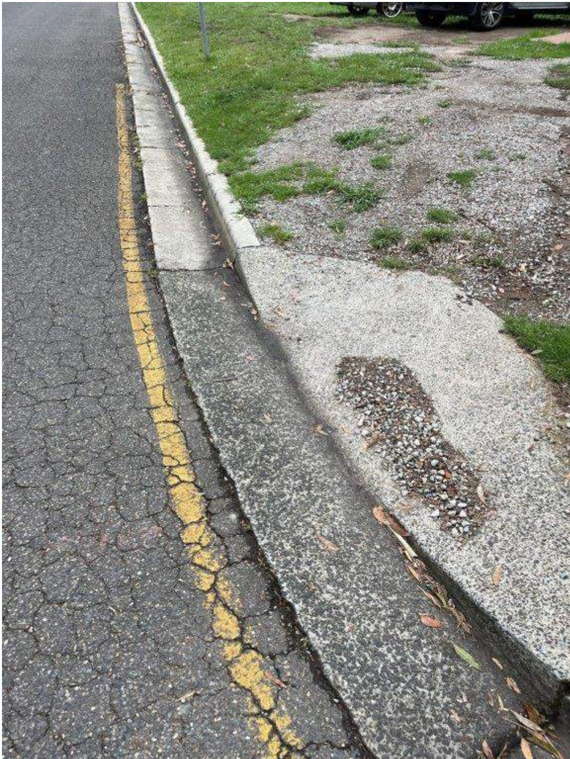
Photo 205 - Taren Point Road - Cracking of pavement
