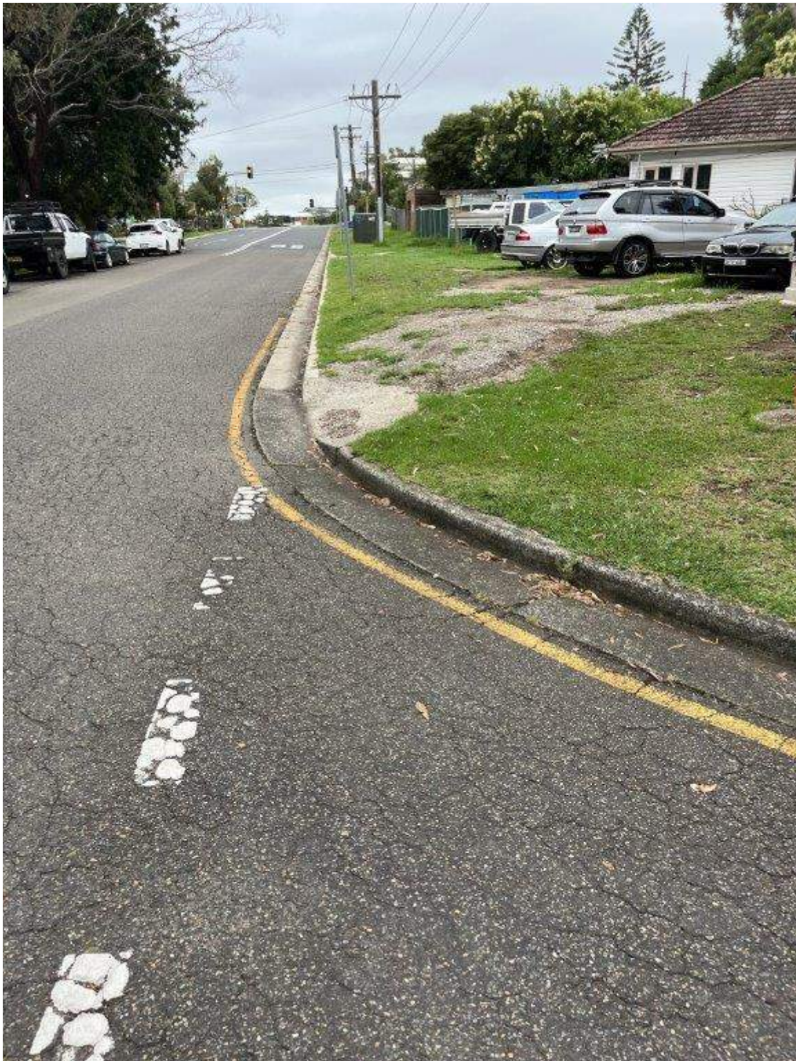
Photo 198 - Taren Point Road - Cracking of pavement
