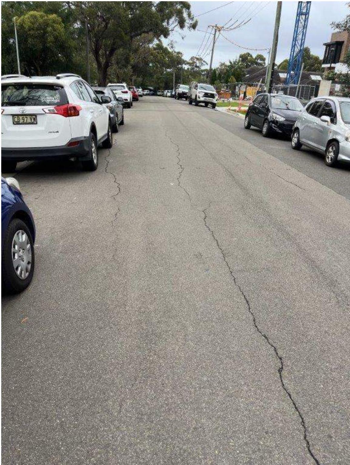
Photo 54 - Hinkler Avenue - Cracking of pavement
