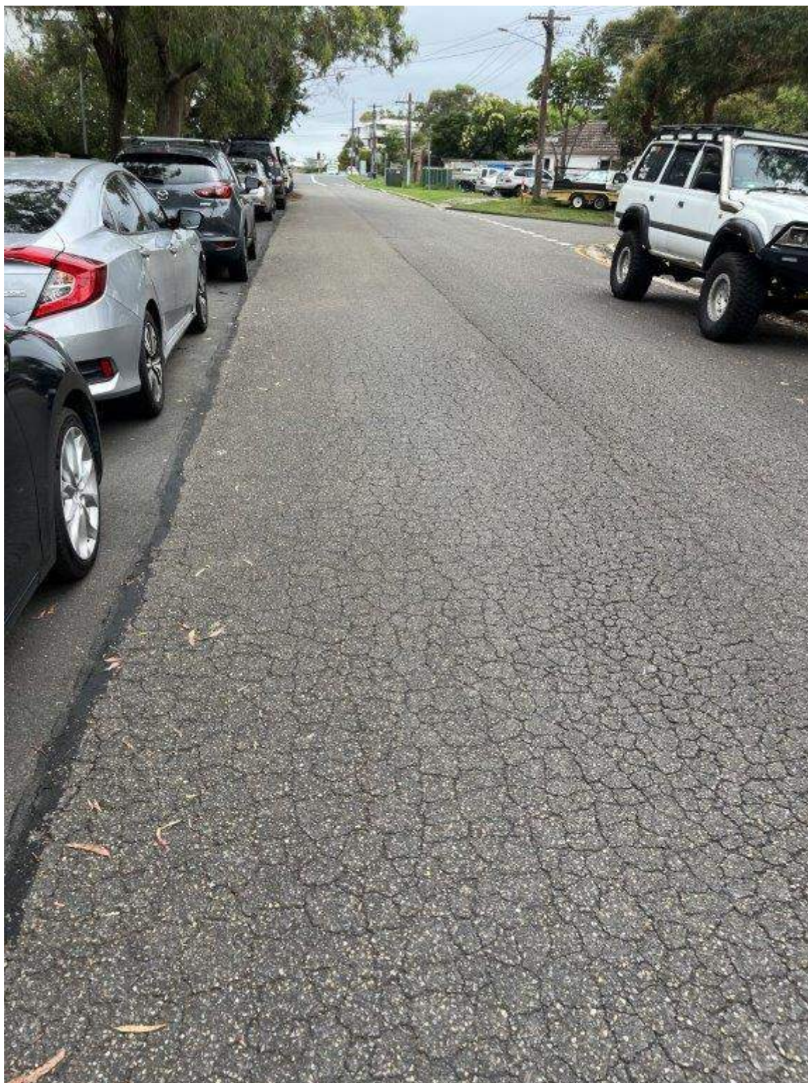
Photo 185 - Taren Point Road - Cracking of pavement
