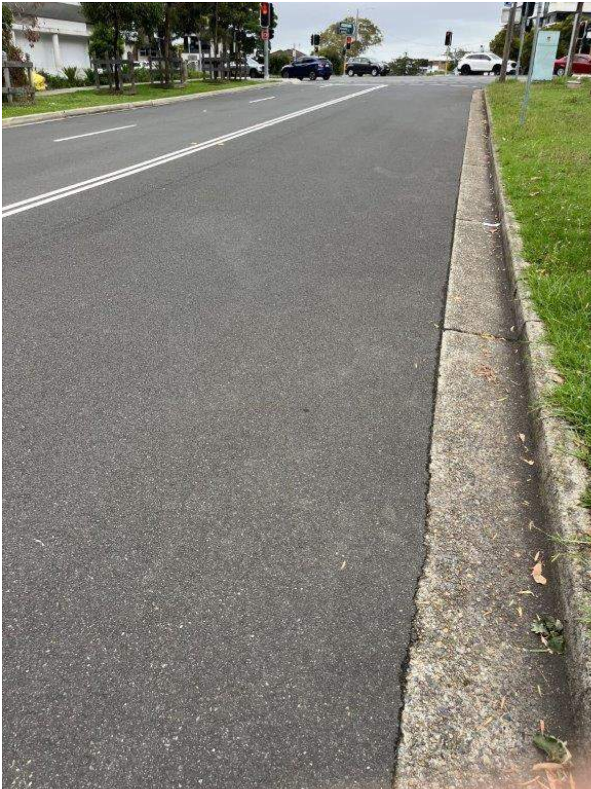
Photo 231 - Taren Point Road - Existing condition of pavement
