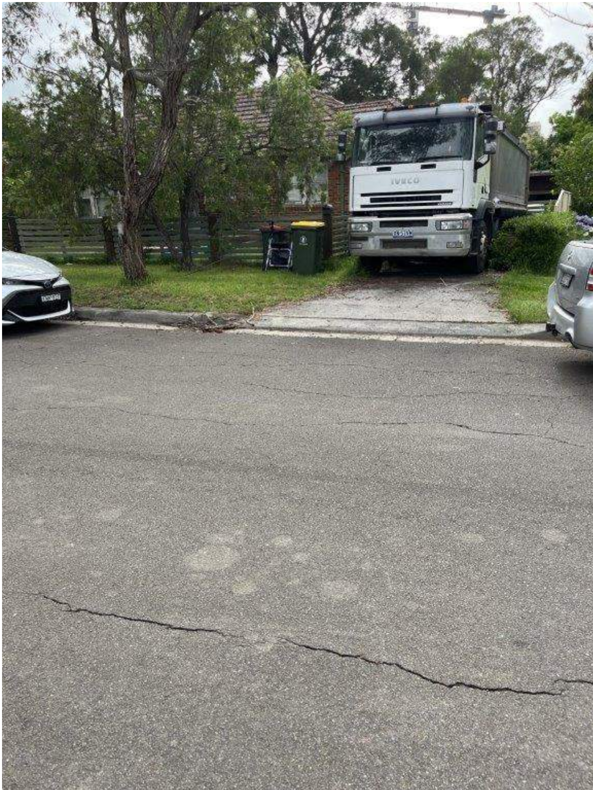
Photo 75 - Hinkler Avenue - Cracking of pavement
