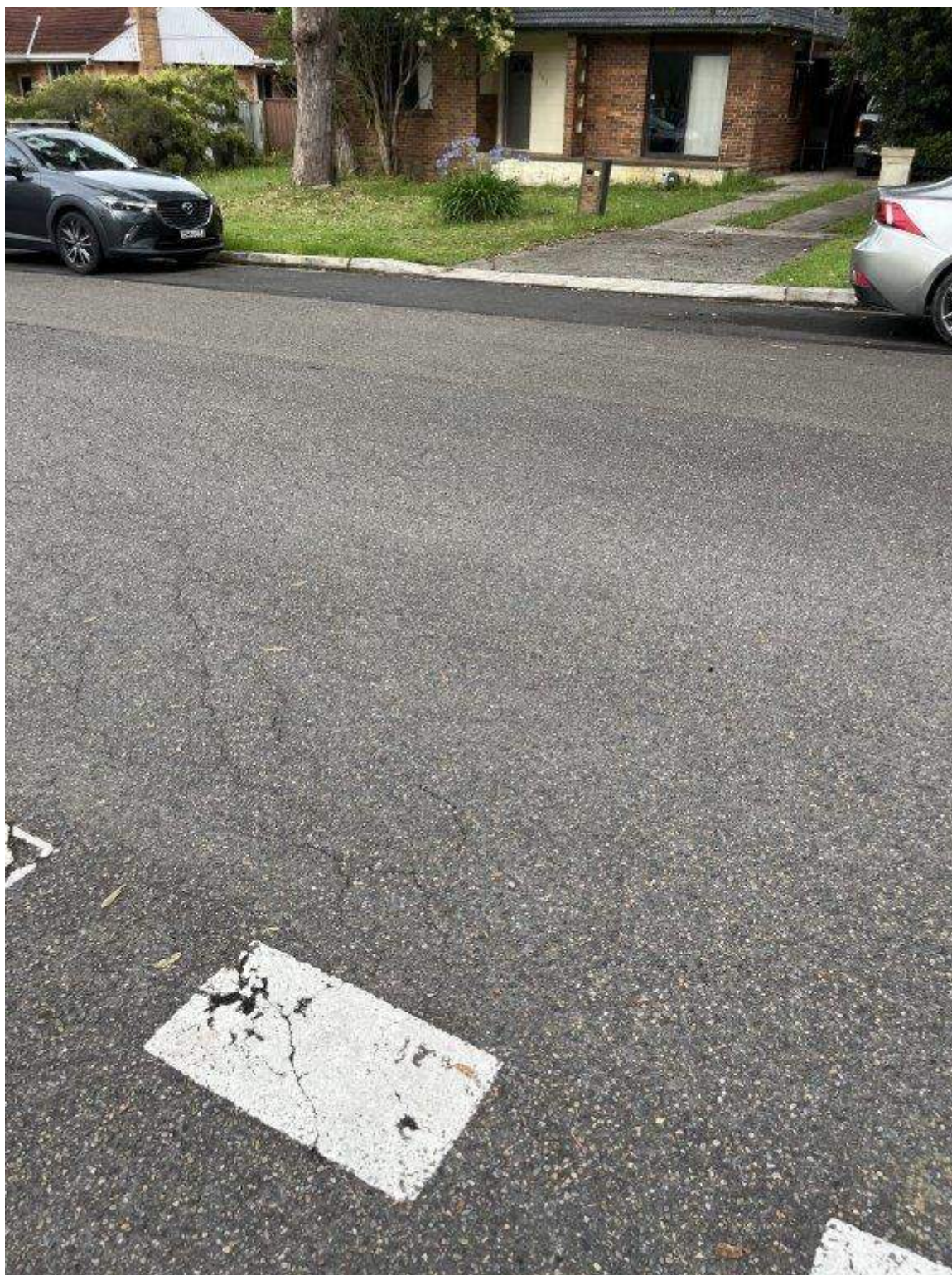
Photo 193 - Taren Point Road - Cracking of pavement
