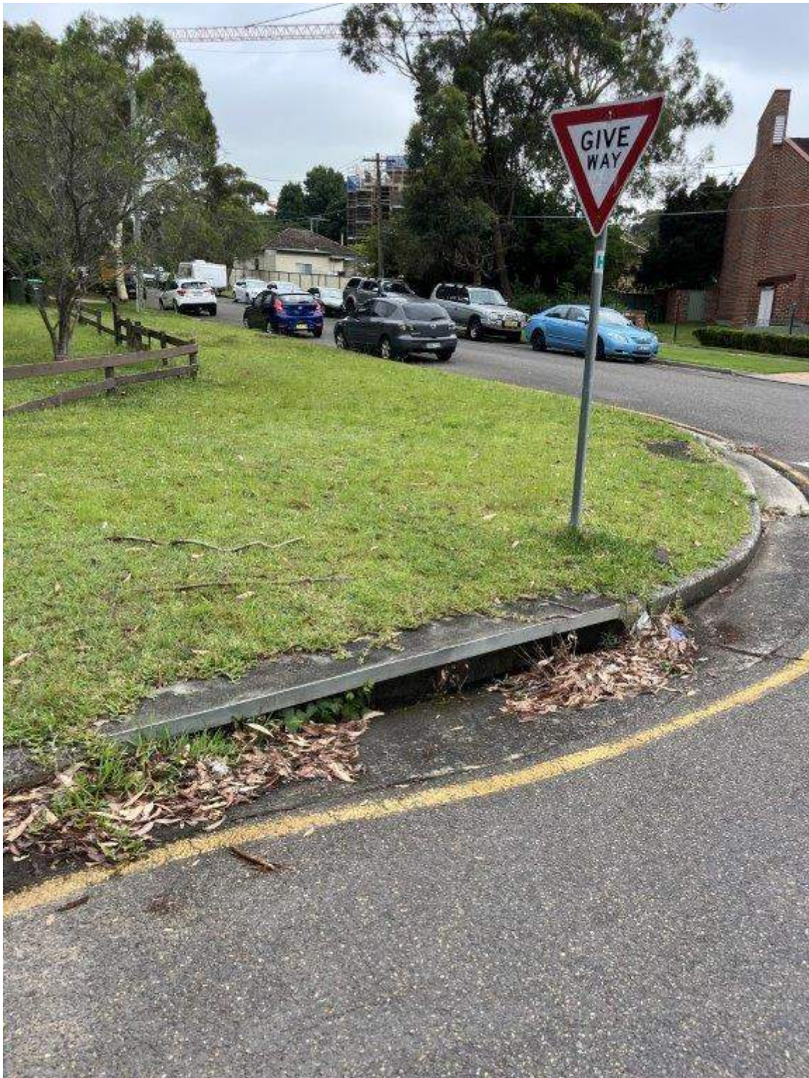
Photo 140 - Hinkler Avenue - Existing condition of signpost
