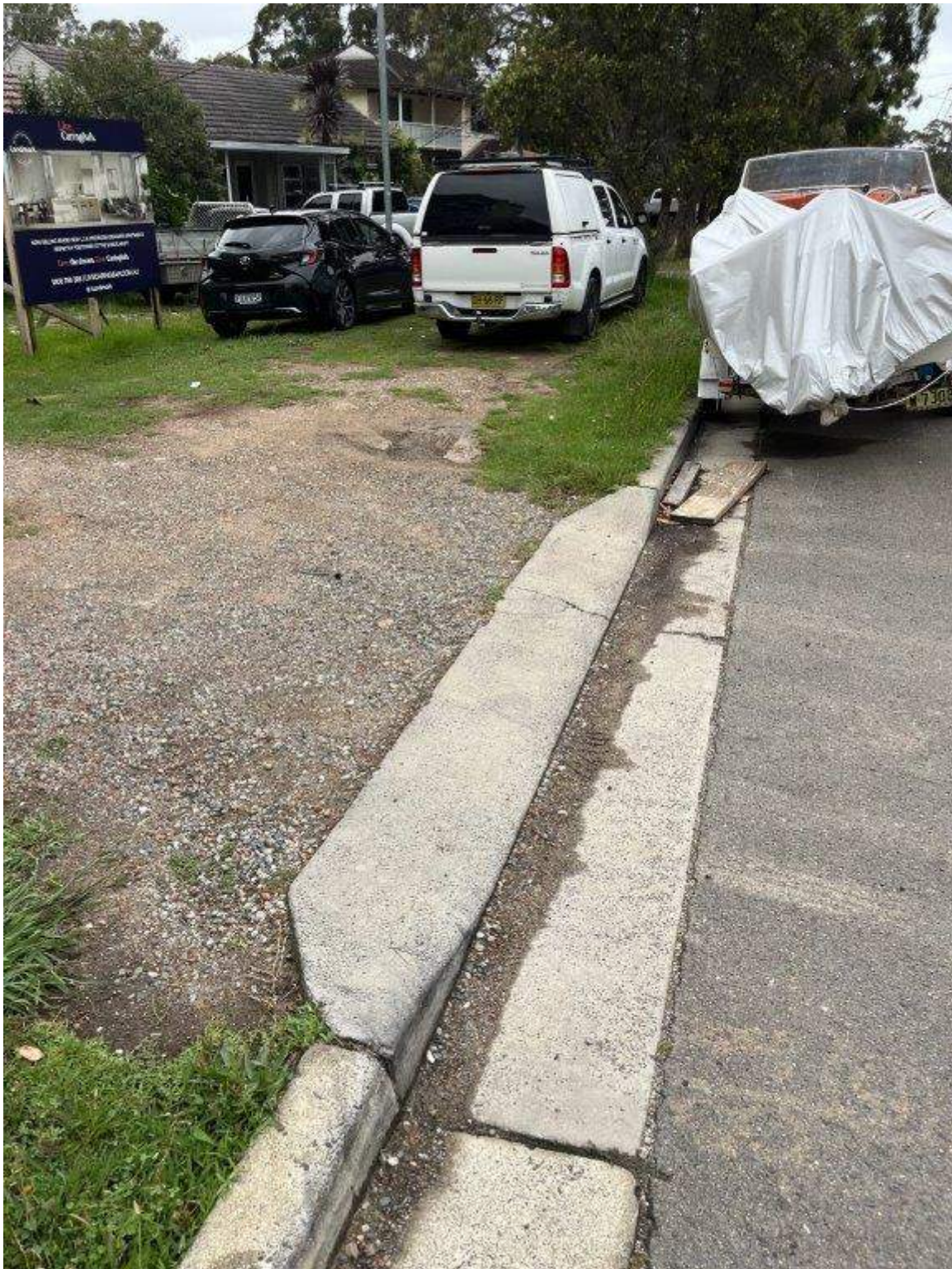
Photo 28 - Hinkler Avenue - Cracking of pavement
