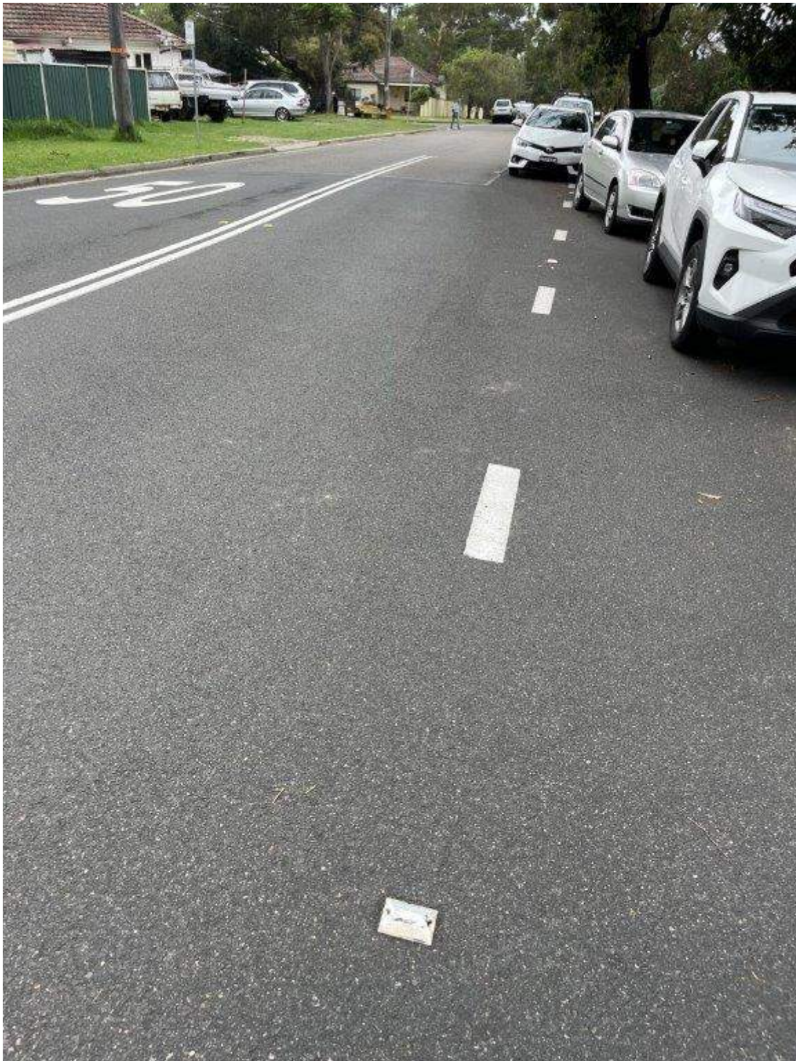
Photo 240 - Taren Point Road - Existing condition of pavement
