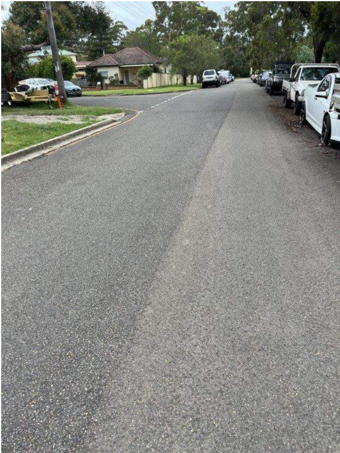
Photo 212 - Taren Point Road - Existing condition of pavement
