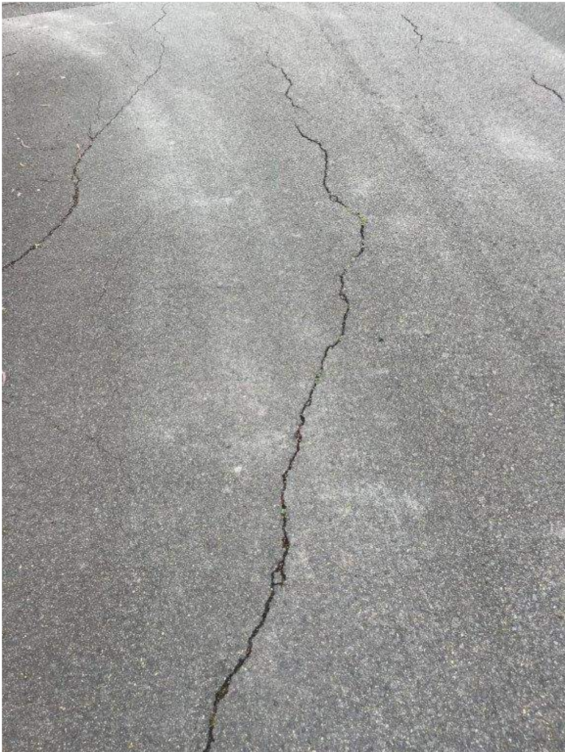
Photo 38 - Hinkler Avenue - Cracking of pavement
