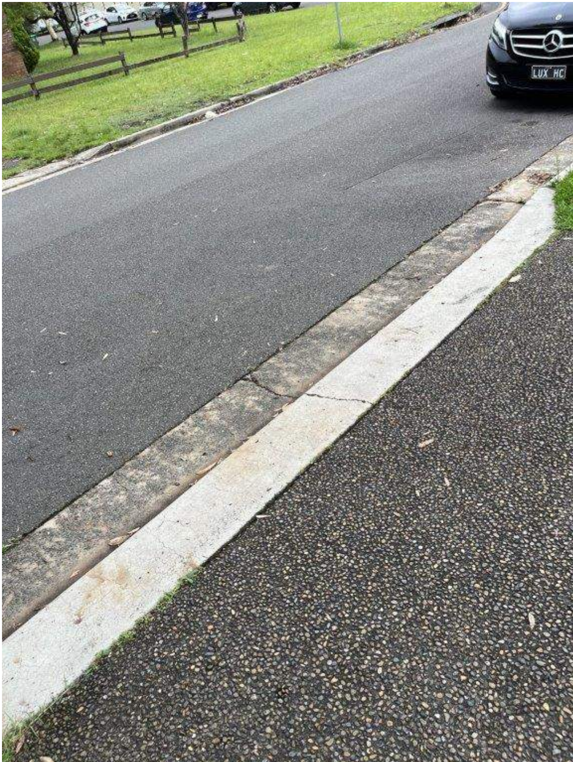
Photo 131 - Hinkler Avenue - Cracking of pavement
