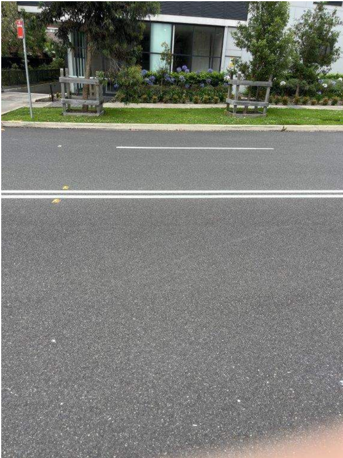
Photo 234 - Taren Point Road - Existing condition of pavement
