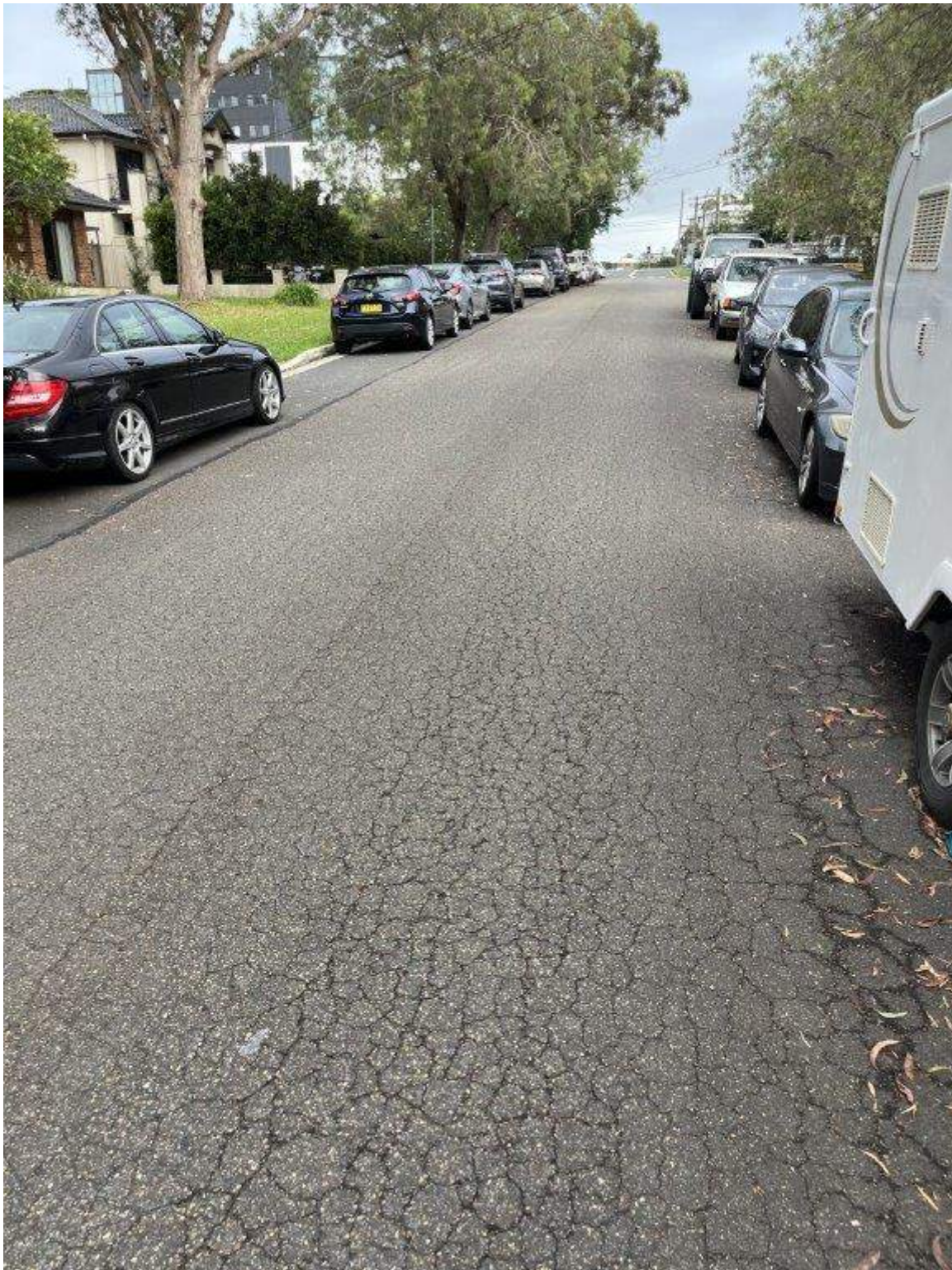
Photo 172 - Taren Point Road - Cracking of pavement
