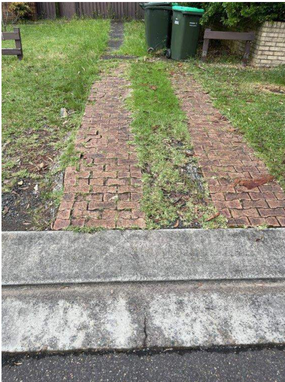
Photo 161 - Taren Point Road - Cracking of pavement
