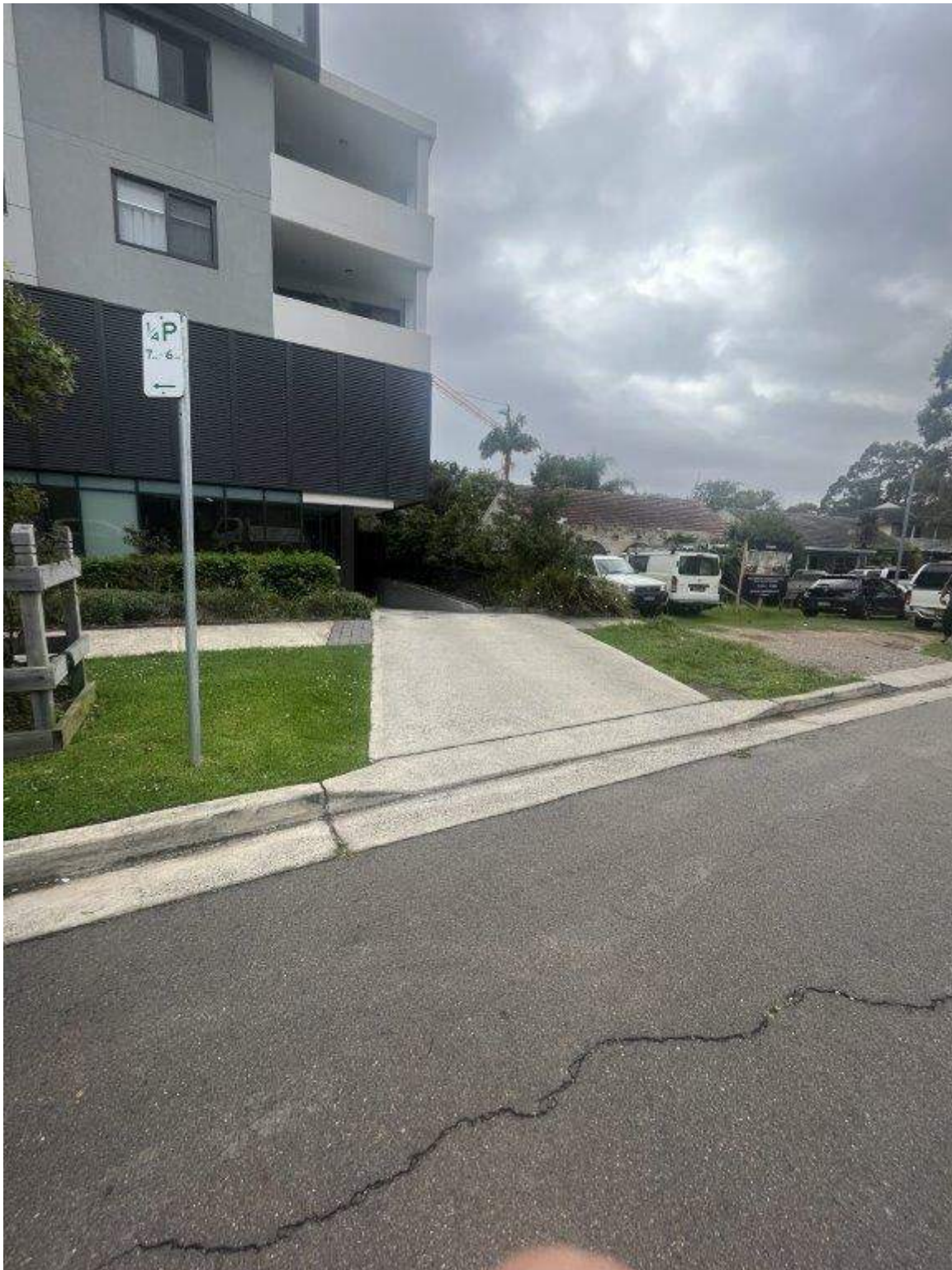
Photo 18 - Hinkler Avenue - Cracking of pavement
