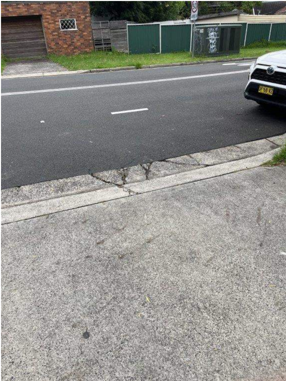
Photo 251 - Taren Point Road - Cracking of pavement
