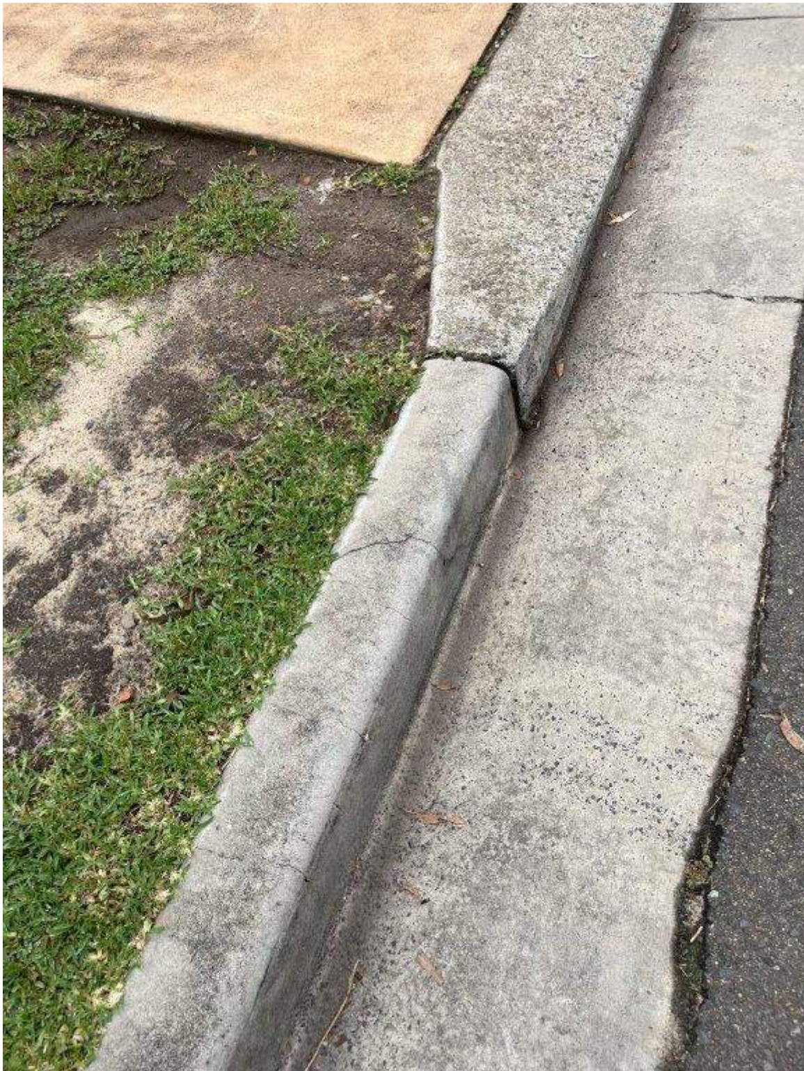
Photo 63 - Hinkler Avenue - Cracking of kerb and pavement
