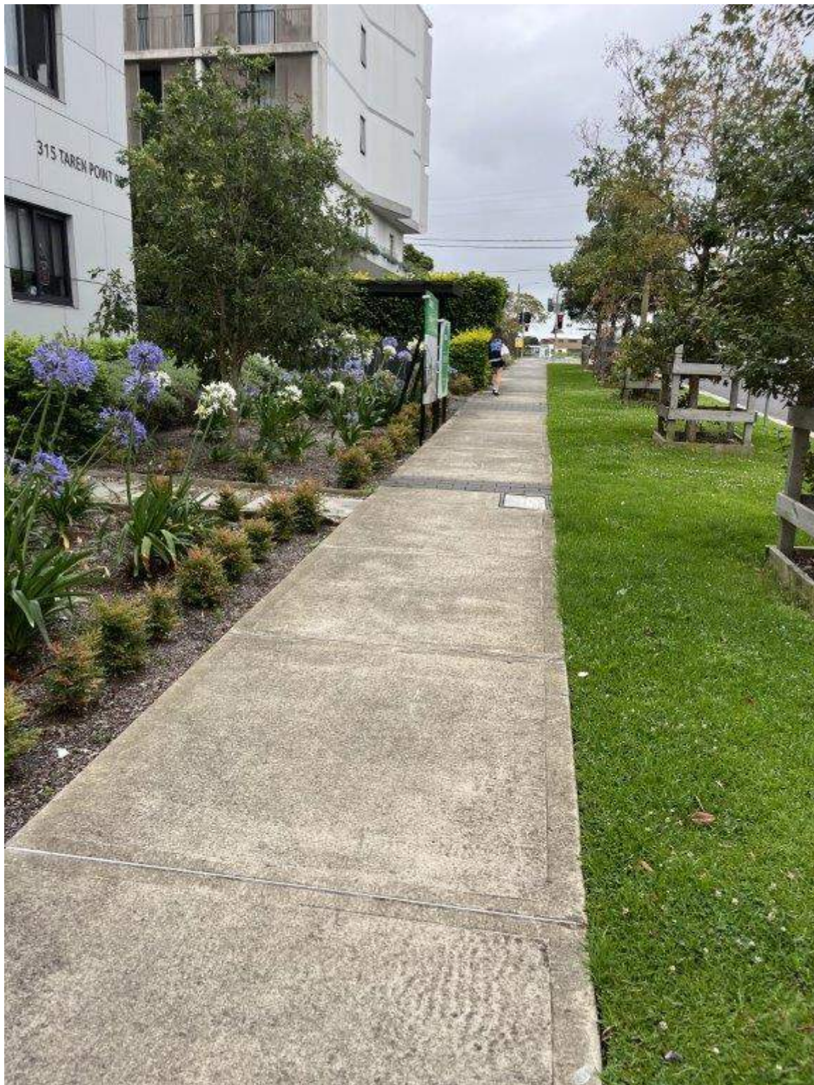
Photo 255 - Taren Point Road - Existing condition of pavement
