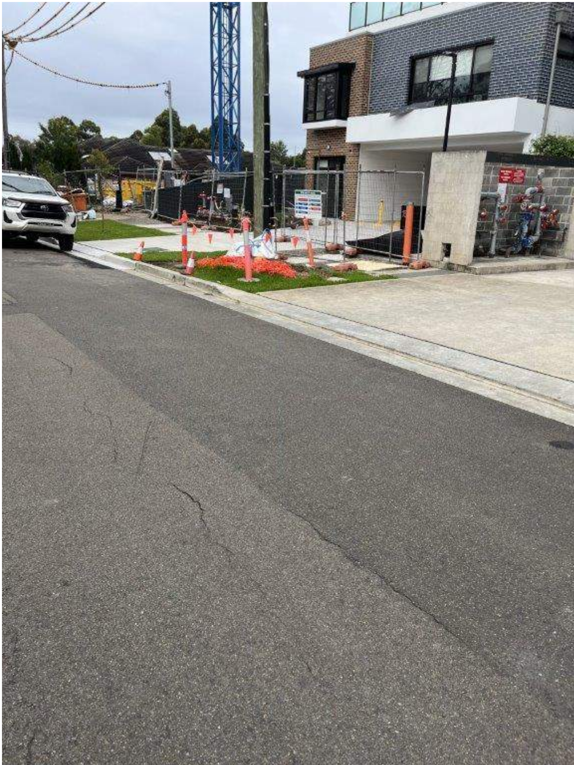
Photo 60 - Hinkler Avenue - Cracking of pavement
