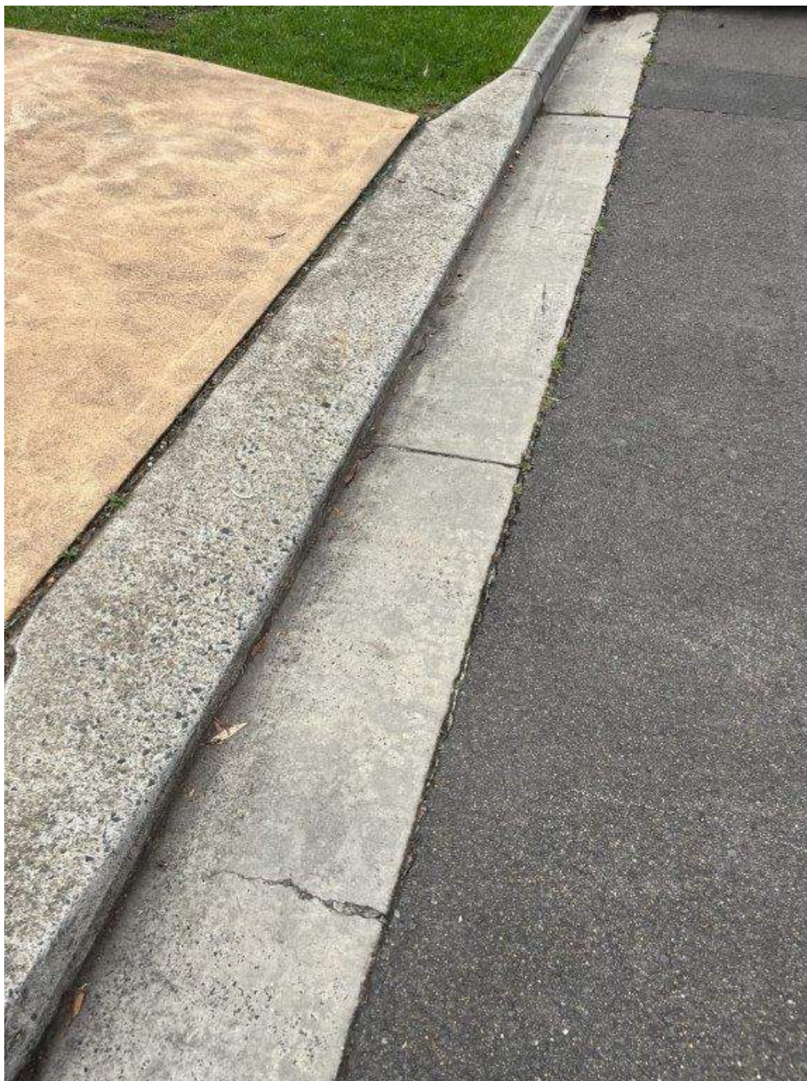
Photo 64 - Hinkler Avenue - Cracking of pavement
