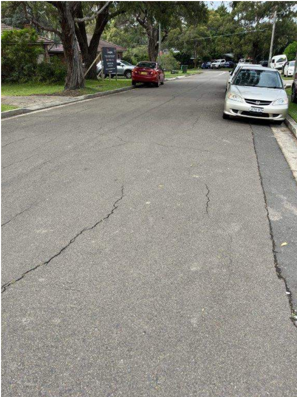
Photo 88 - Hinkler Avenue - Cracking of pavement
