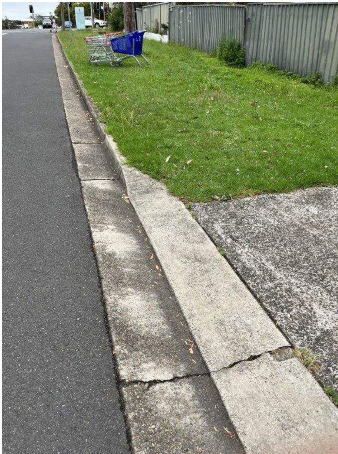
Photo 228 - Taren Point Road - Cracking of pavement
