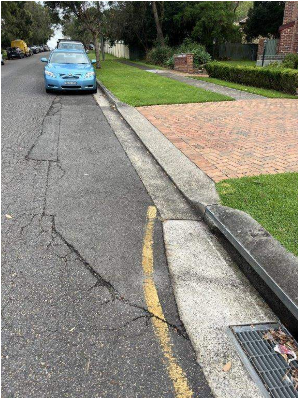
Photo 145 - Taren Point Road - Cracking of pavement
