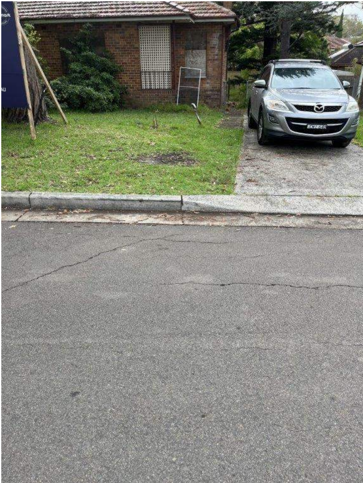
Photo 100 - Hinkler Avenue - Cracking of pavement
