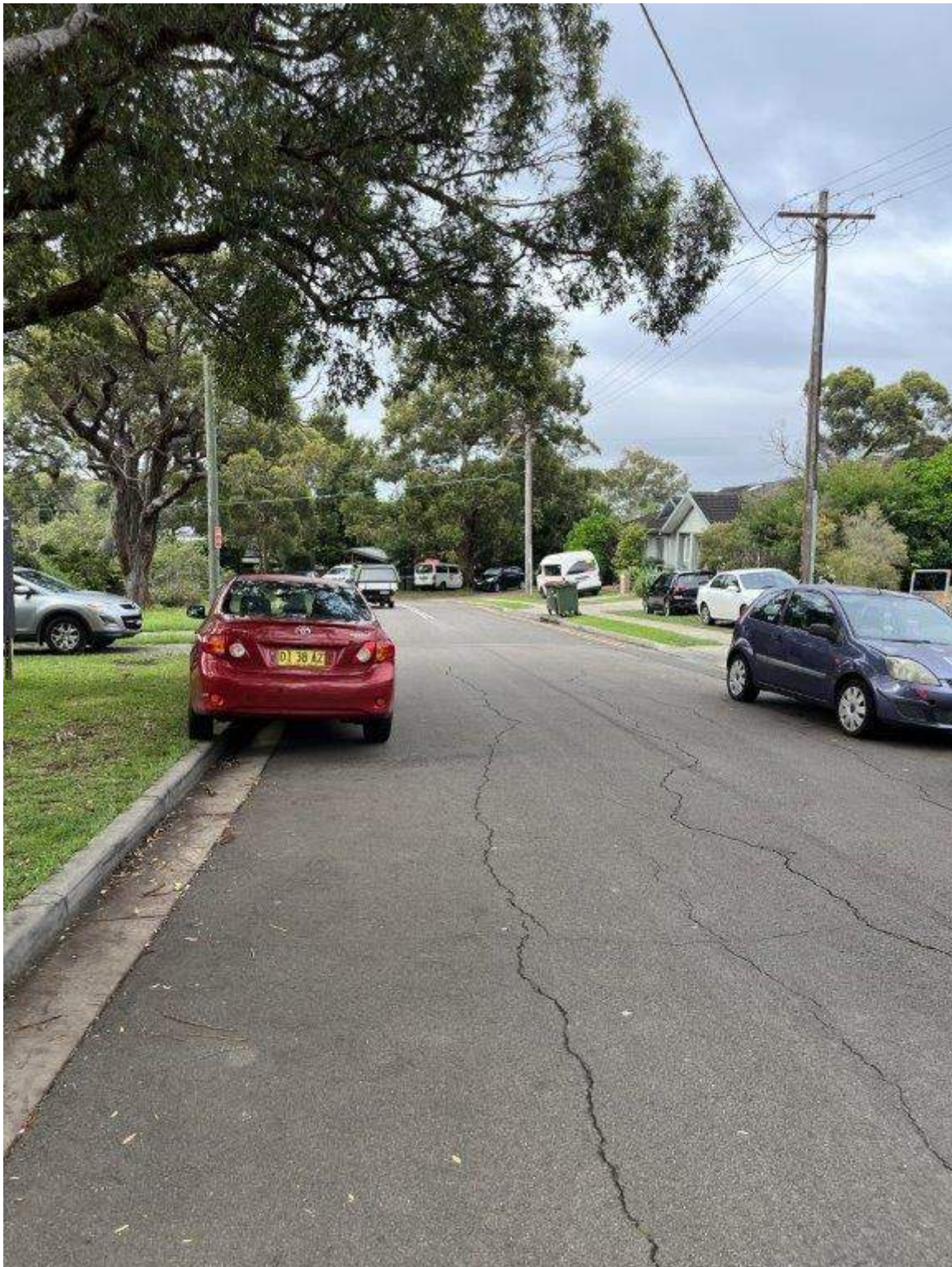
Photo 94 - Hinkler Avenue - Cracking of pavement
