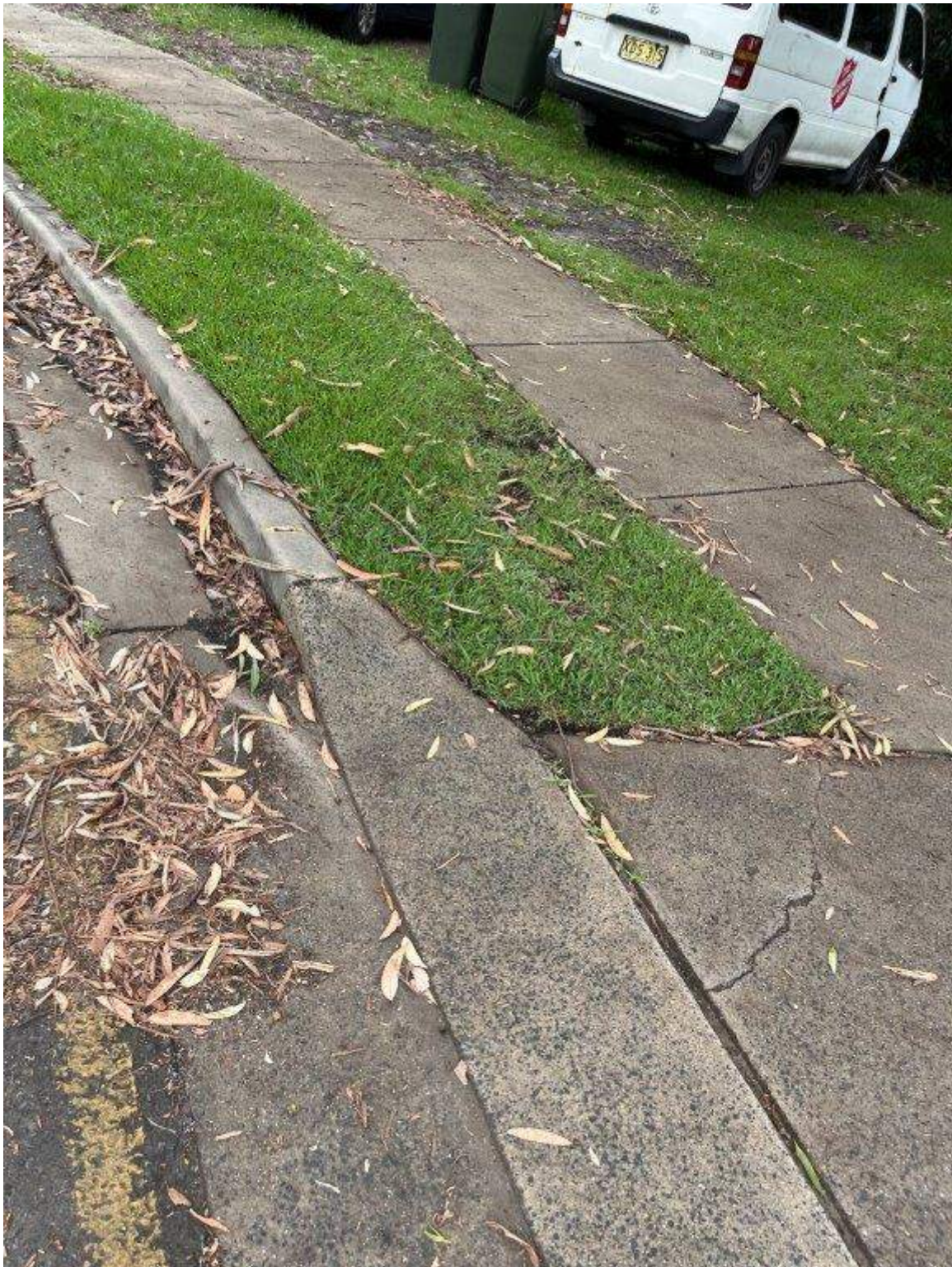
Photo 110 - Hinkler Avenue - Cracking of pavement
