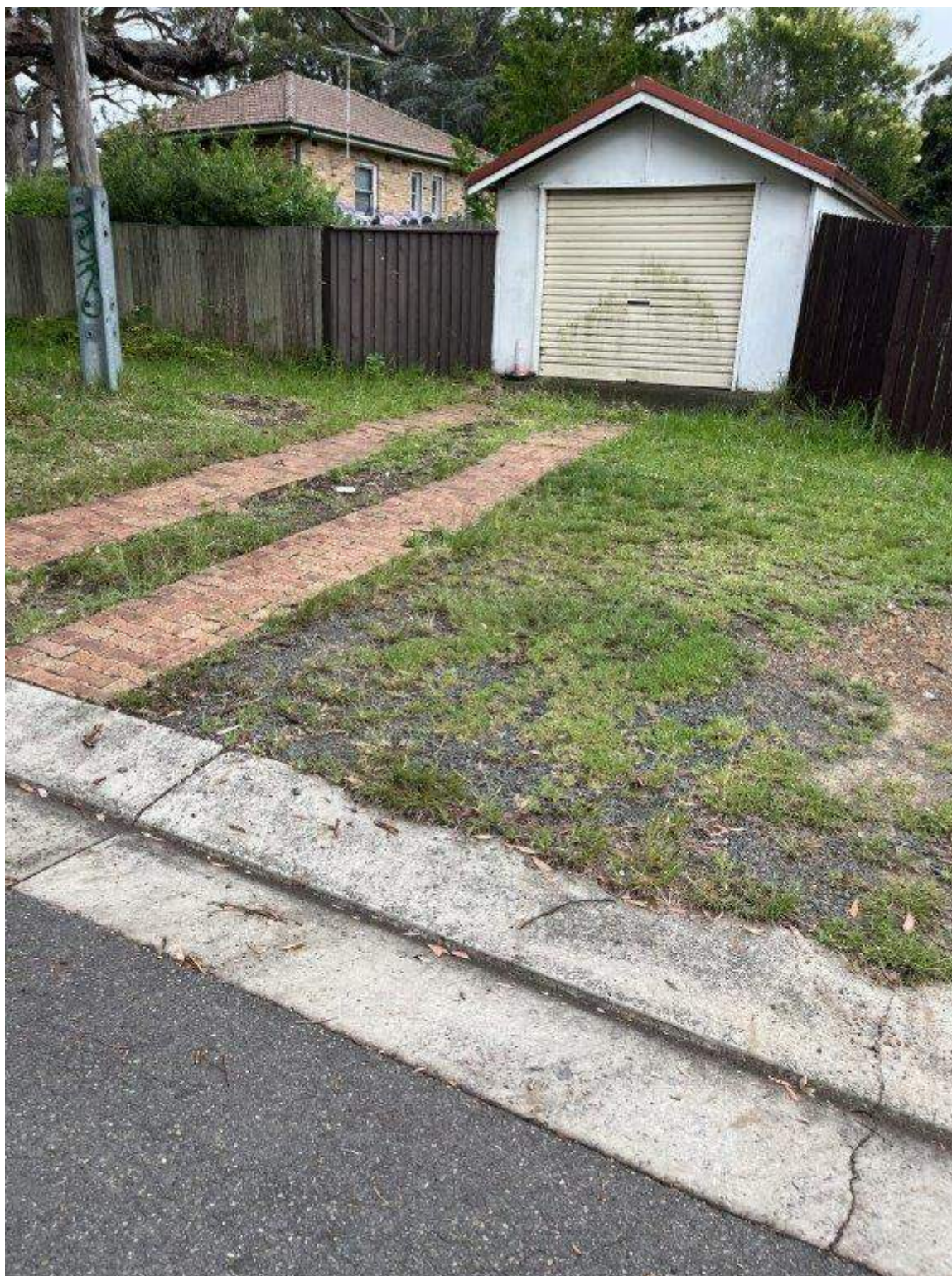
Photo 133 - Hinkler Avenue - Cracking of pavement
