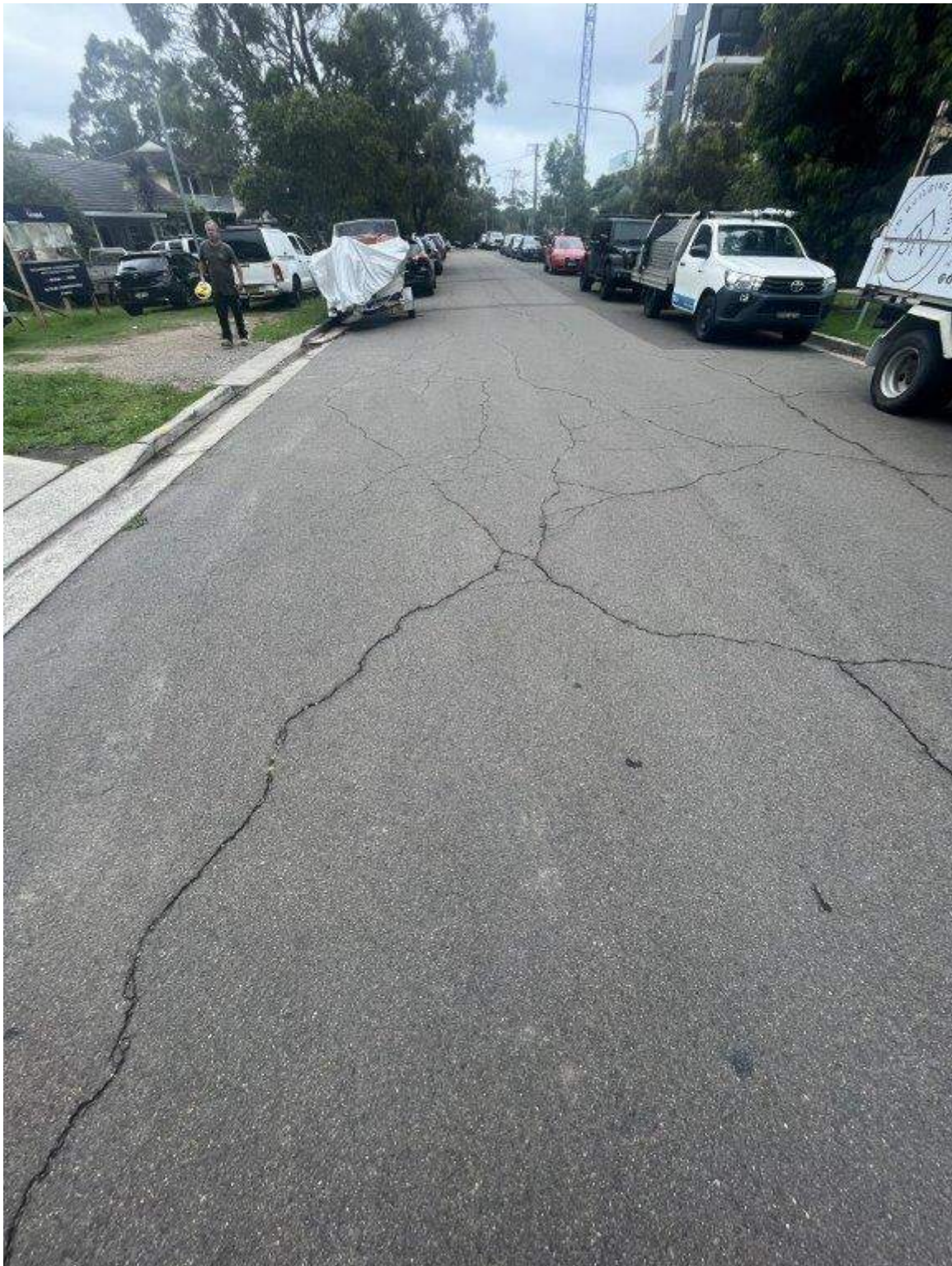
Photo 19 - Hinkler Avenue - Cracking of pavement
