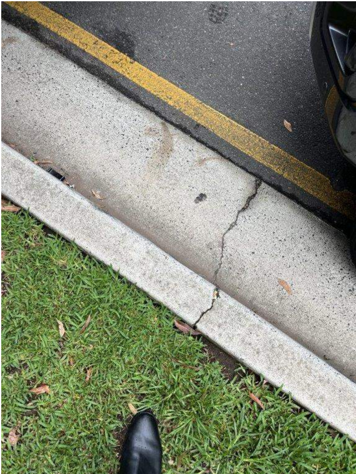
Photo 7 - Hinkler Avenue - Cracking of kerb and pavement
