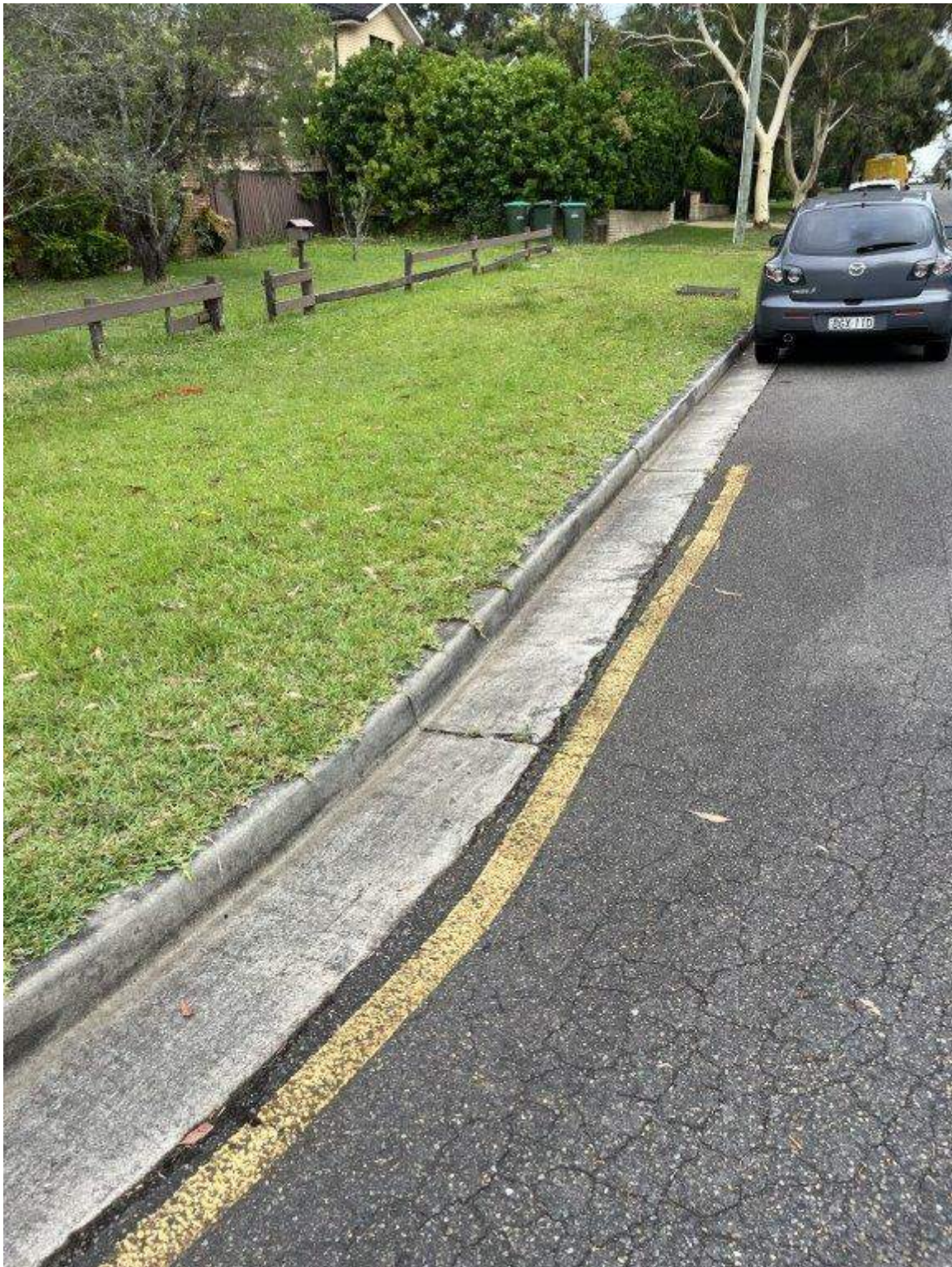
Photo 150 - Taren Point Road - Cracking of pavement
