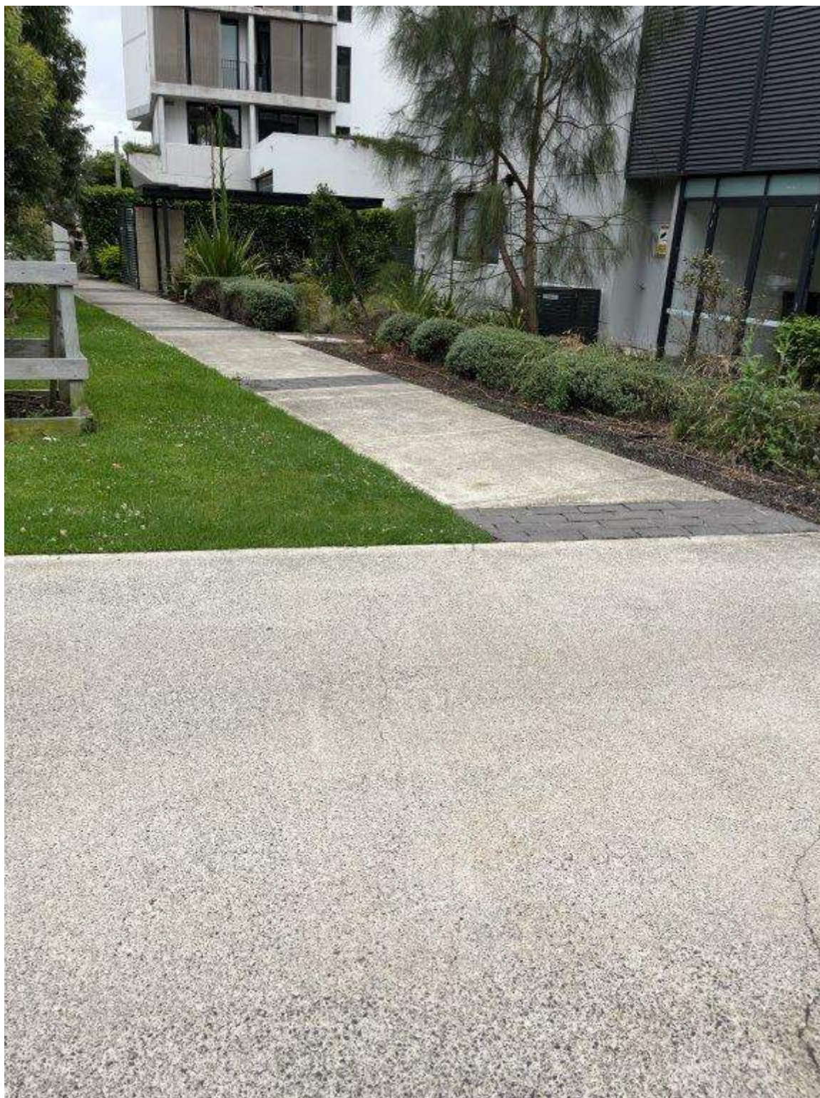
Photo 23 - Hinkler Avenue - Cracking of pavement
