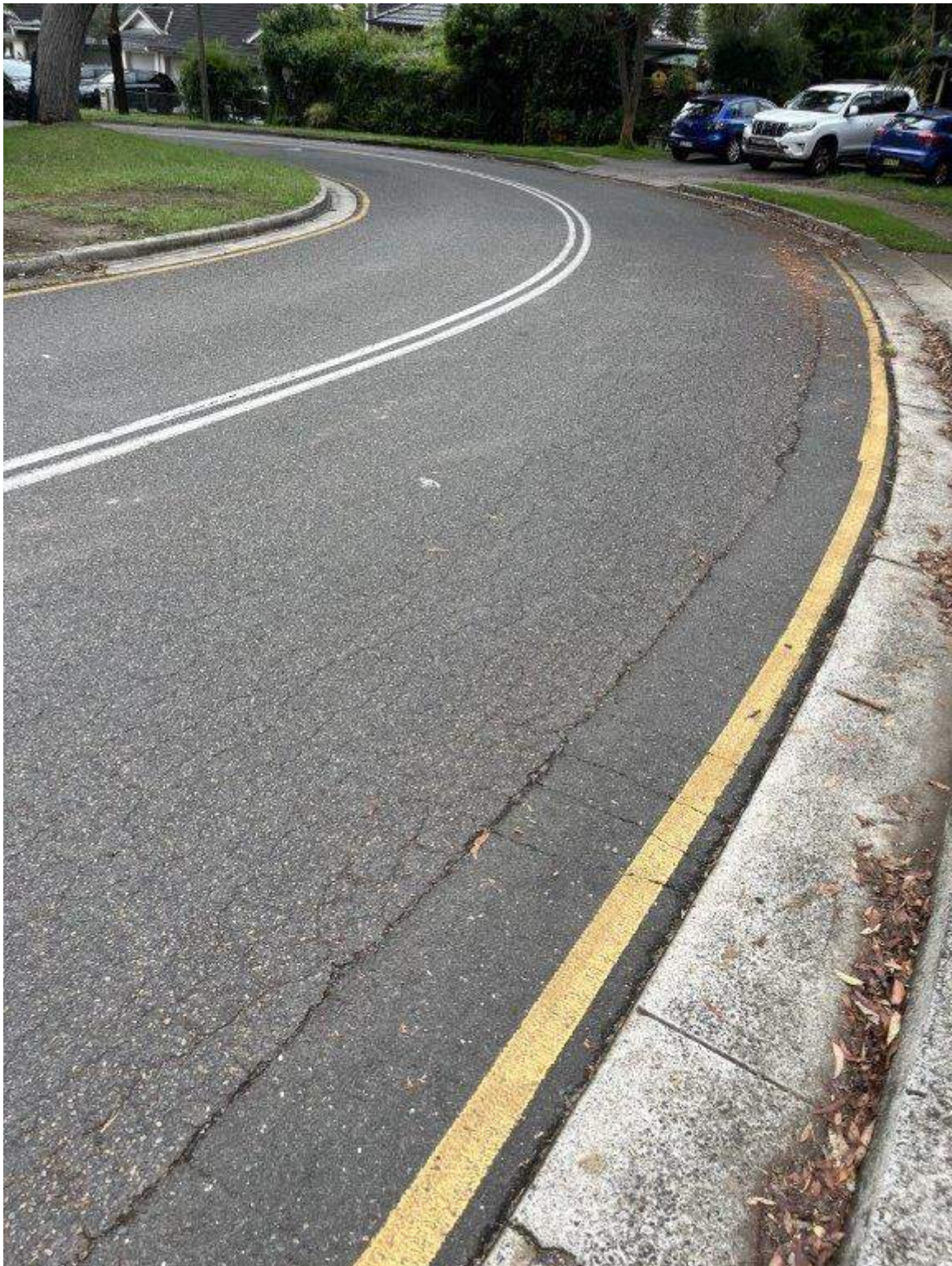
Photo 108 - Hinkler Avenue - Cracking of pavement
