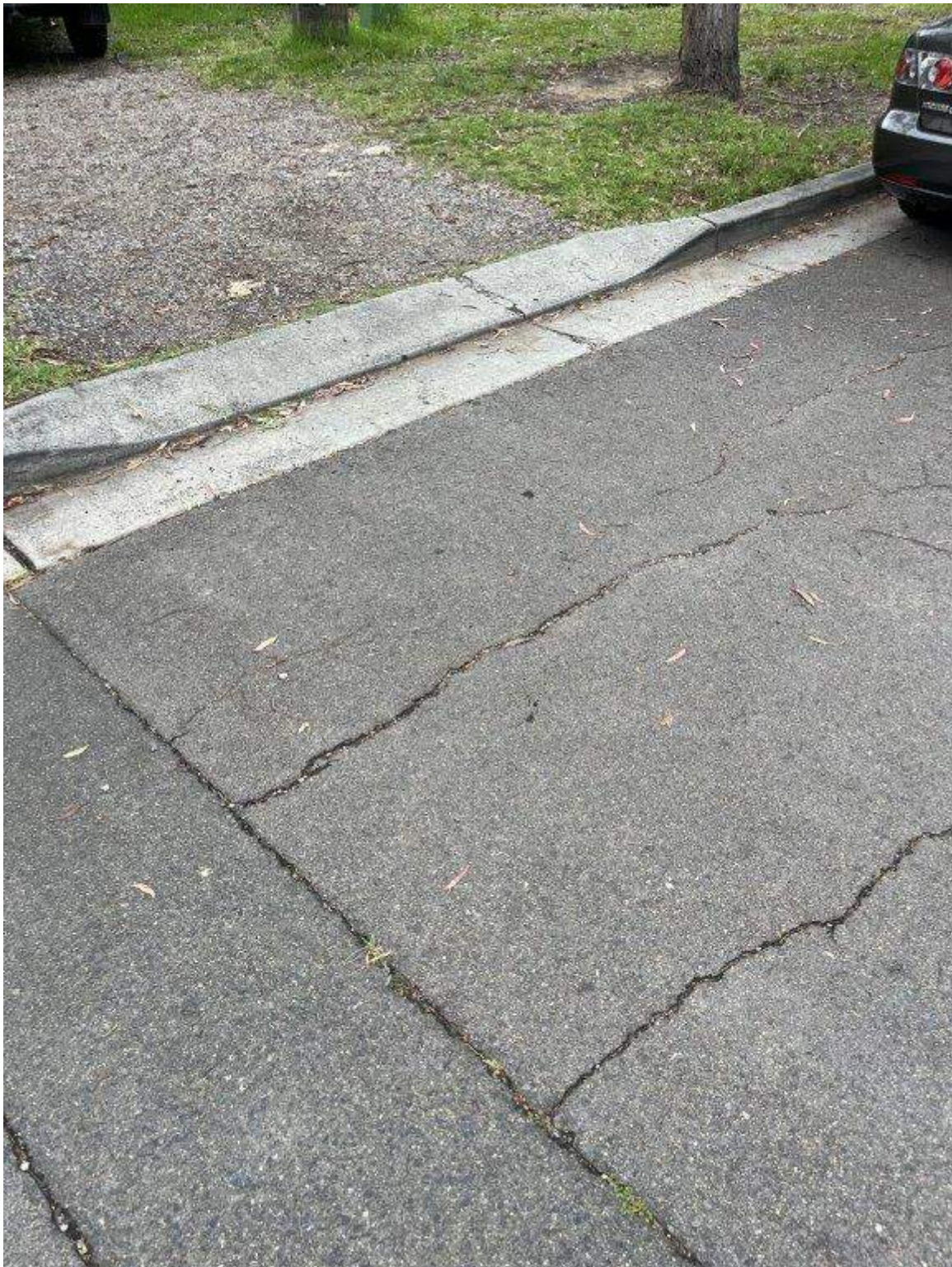
Photo 34 - Hinkler Avenue - Cracking of pavement
