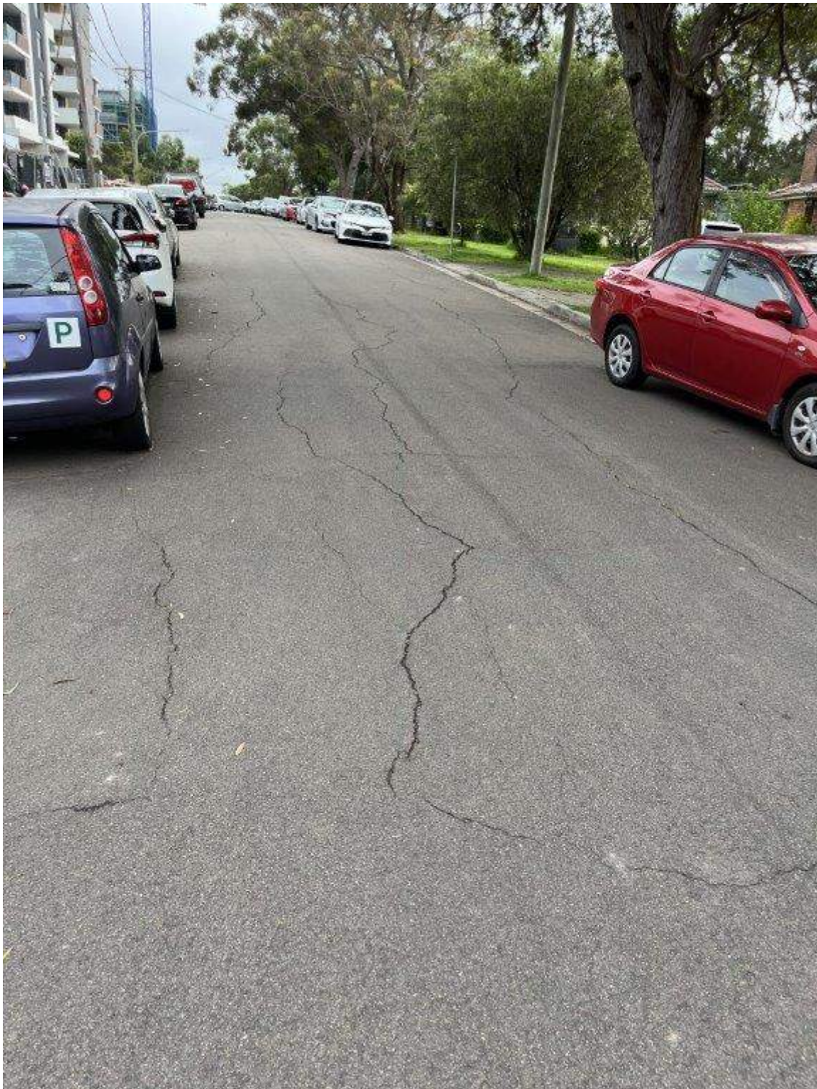
Photo 99 - Hinkler Avenue - Cracking of pavement
