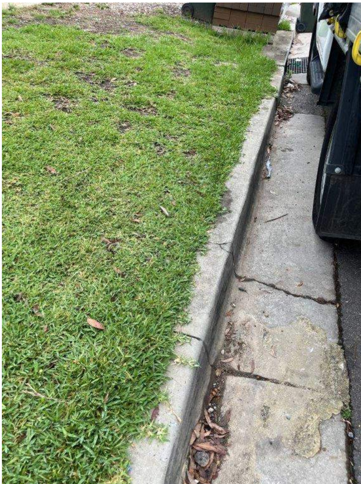
Photo 80 - Hinkler Avenue - Cracking of kerb and pavement
