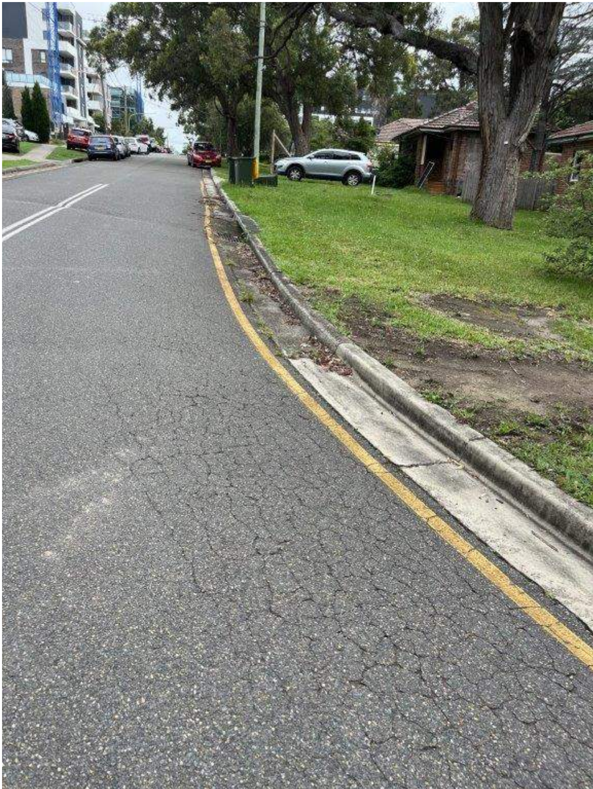
Photo 115 - Hinkler Avenue - Cracking of pavement
