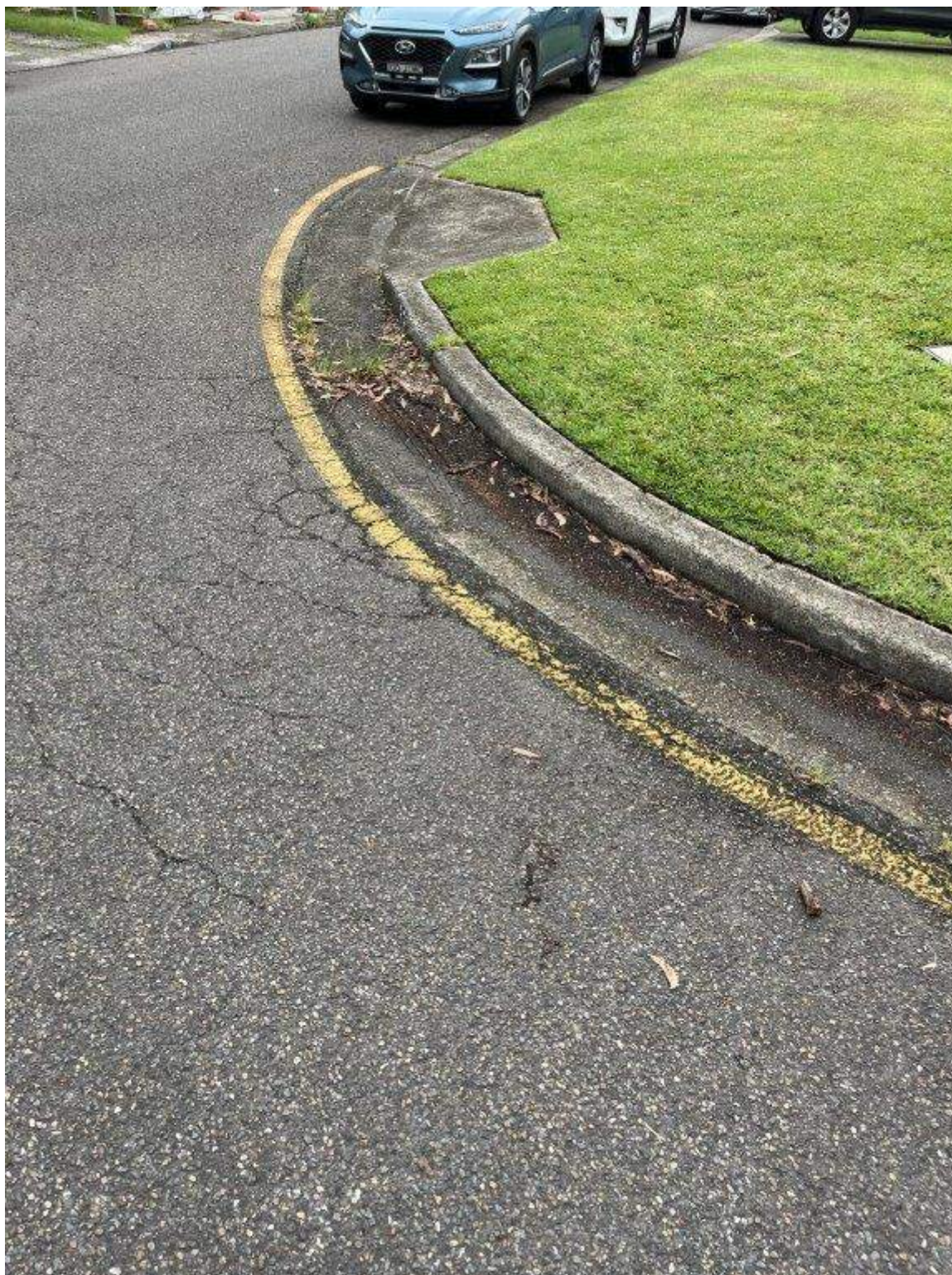
Photo 189 - Taren Point Road - Cracking of pavement
