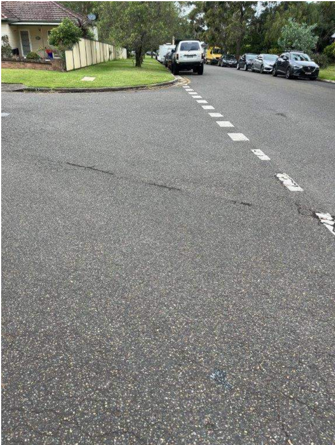
Photo 202 - Taren Point Road - Cracking of pavement
