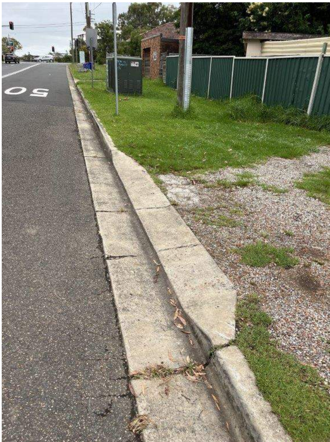
Photo 217 - Taren Point Road - Cracking of pavement
