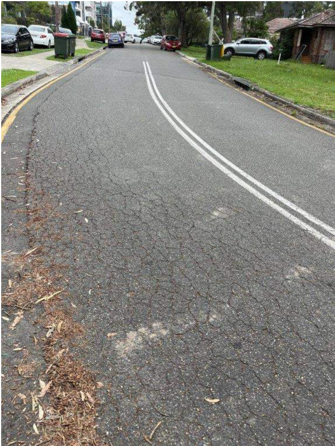
Photo 114 - Hinkler Avenue - Cracking of pavement
