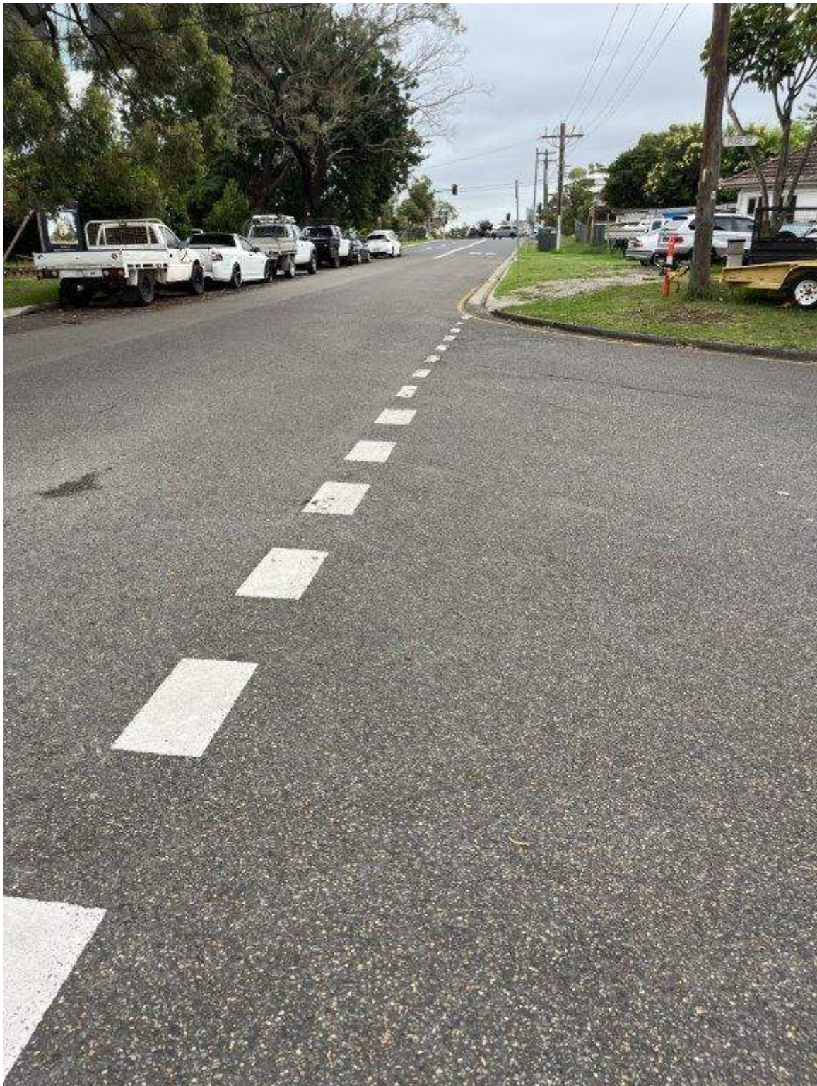
Photo 186 - Taren Point Road - Existing condition of pavement
