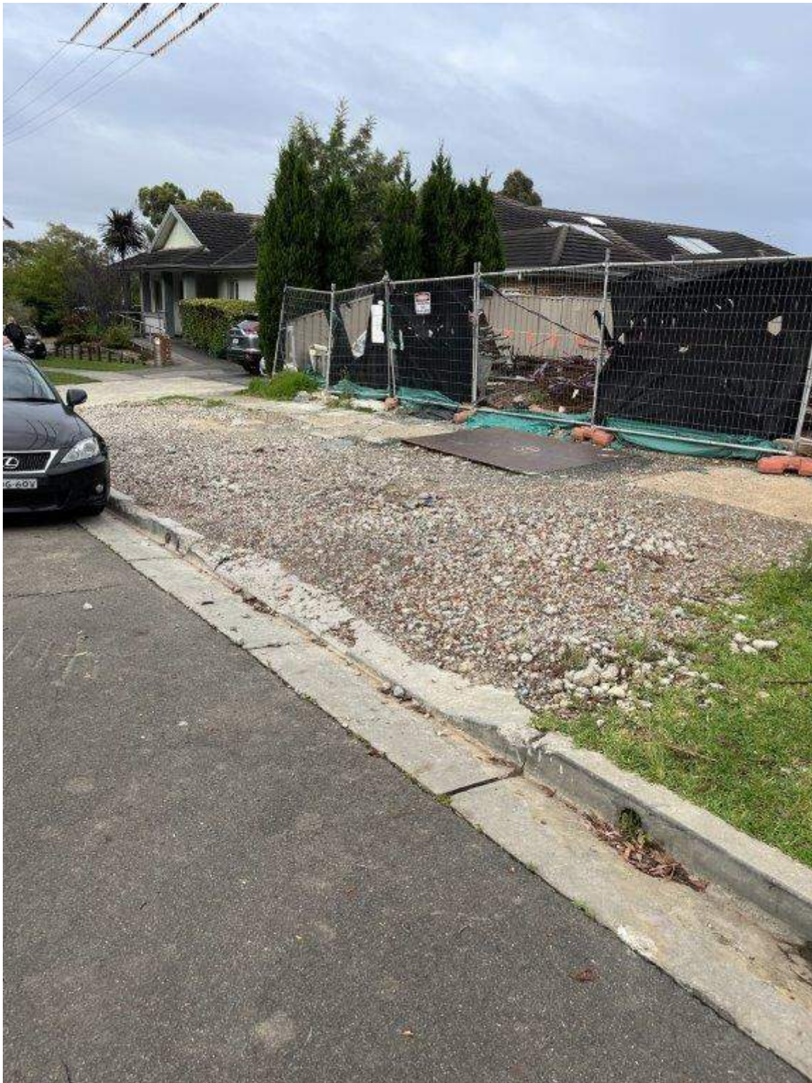
Photo 77 - Hinkler Avenue - Cracking of pavement
