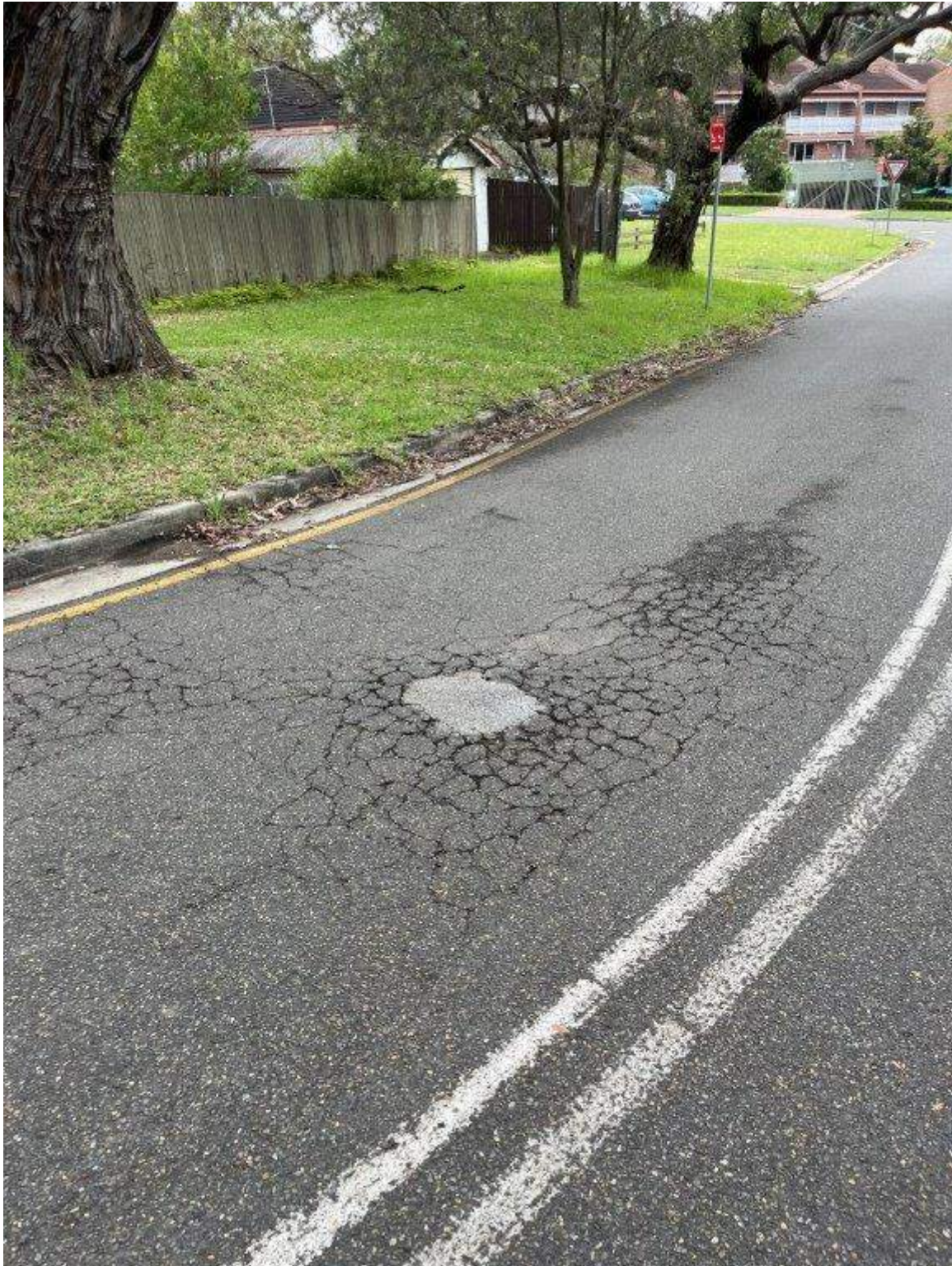
Photo 121 - Hinkler Avenue - Cracking of pavement and patching
