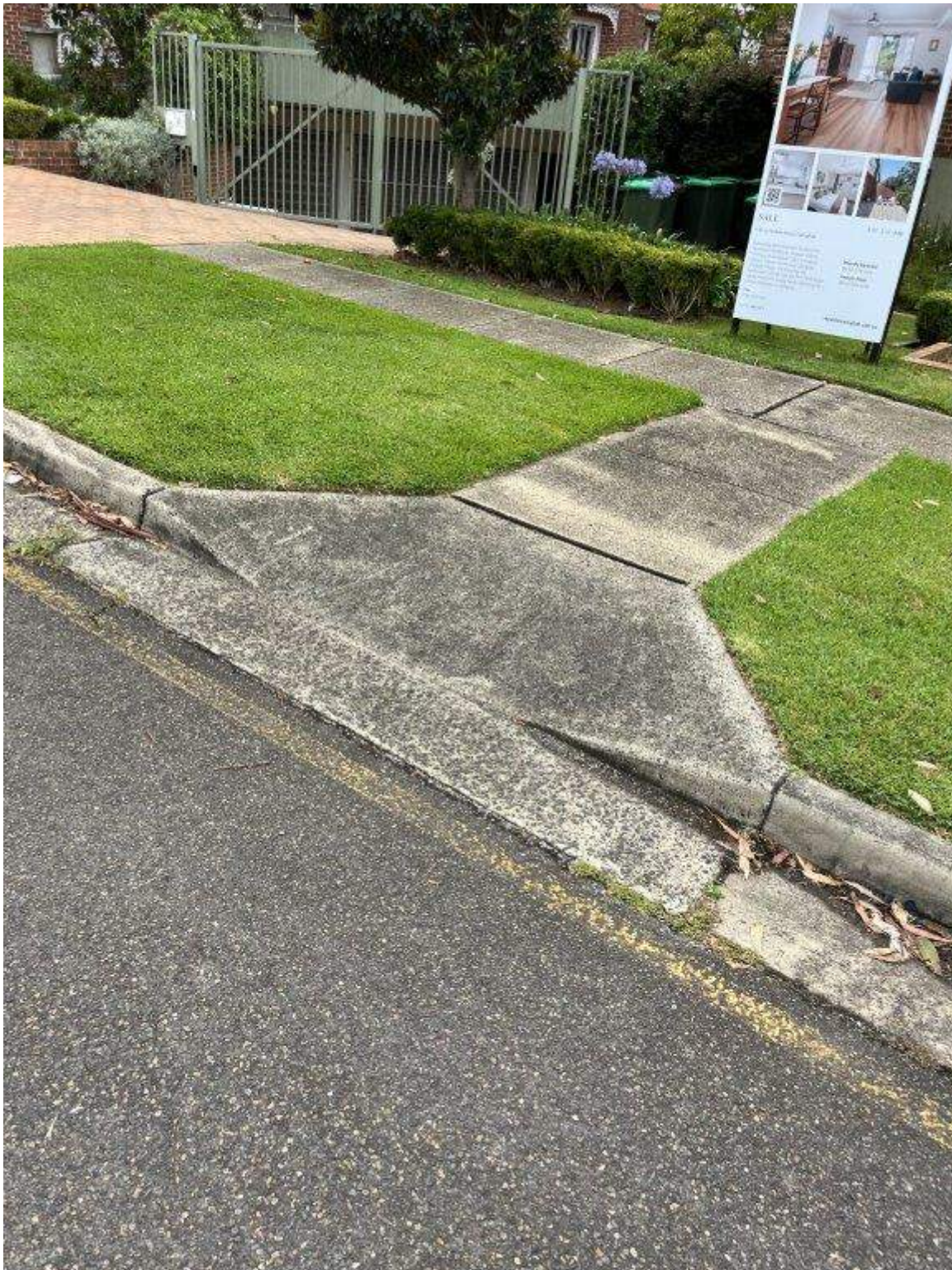
Photo 143 - Taren Point Road - Existing condition of pavement
