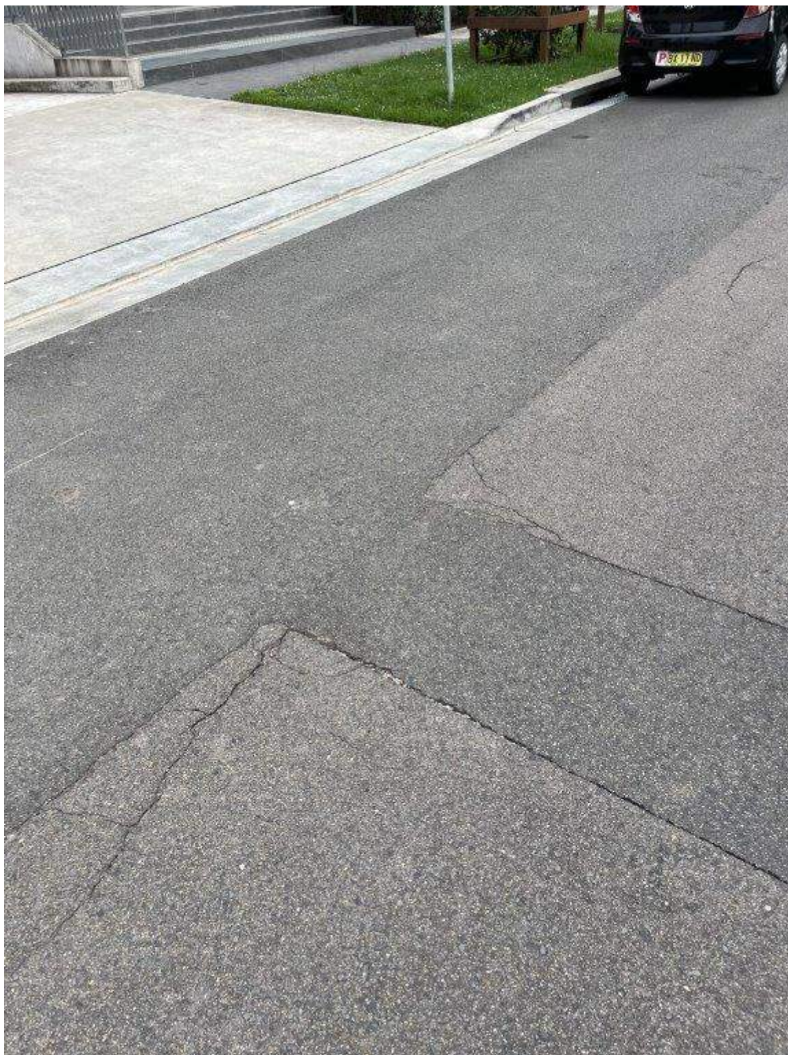
Photo 68 - Hinkler Avenue - Cracking of pavement
