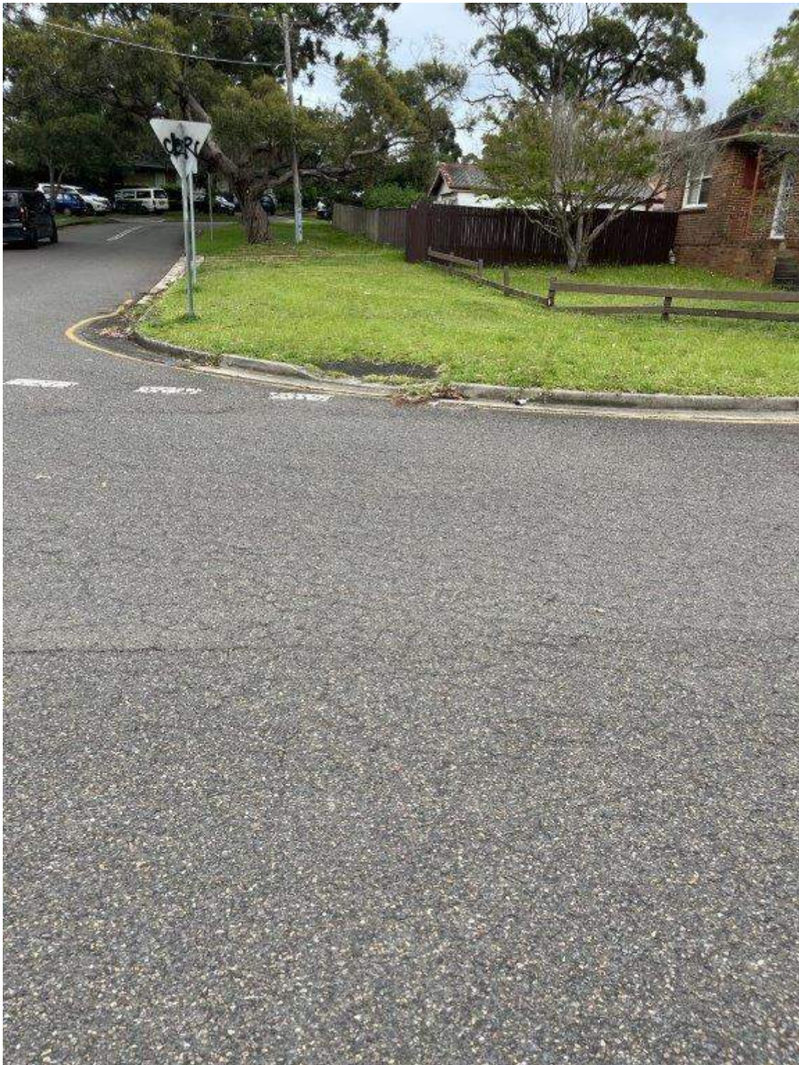
Photo 148 - Taren Point Road - Existing condition of pavement
