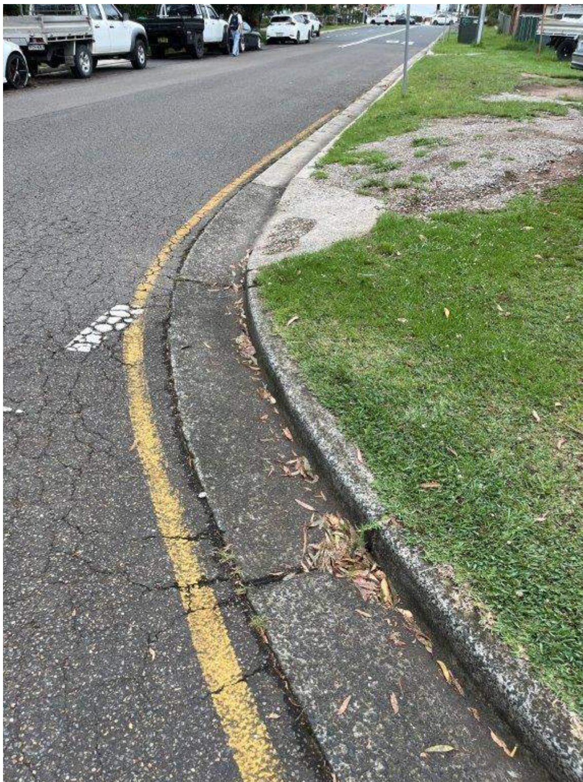
Photo 204 - Taren Point Road - Cracking of pavement
