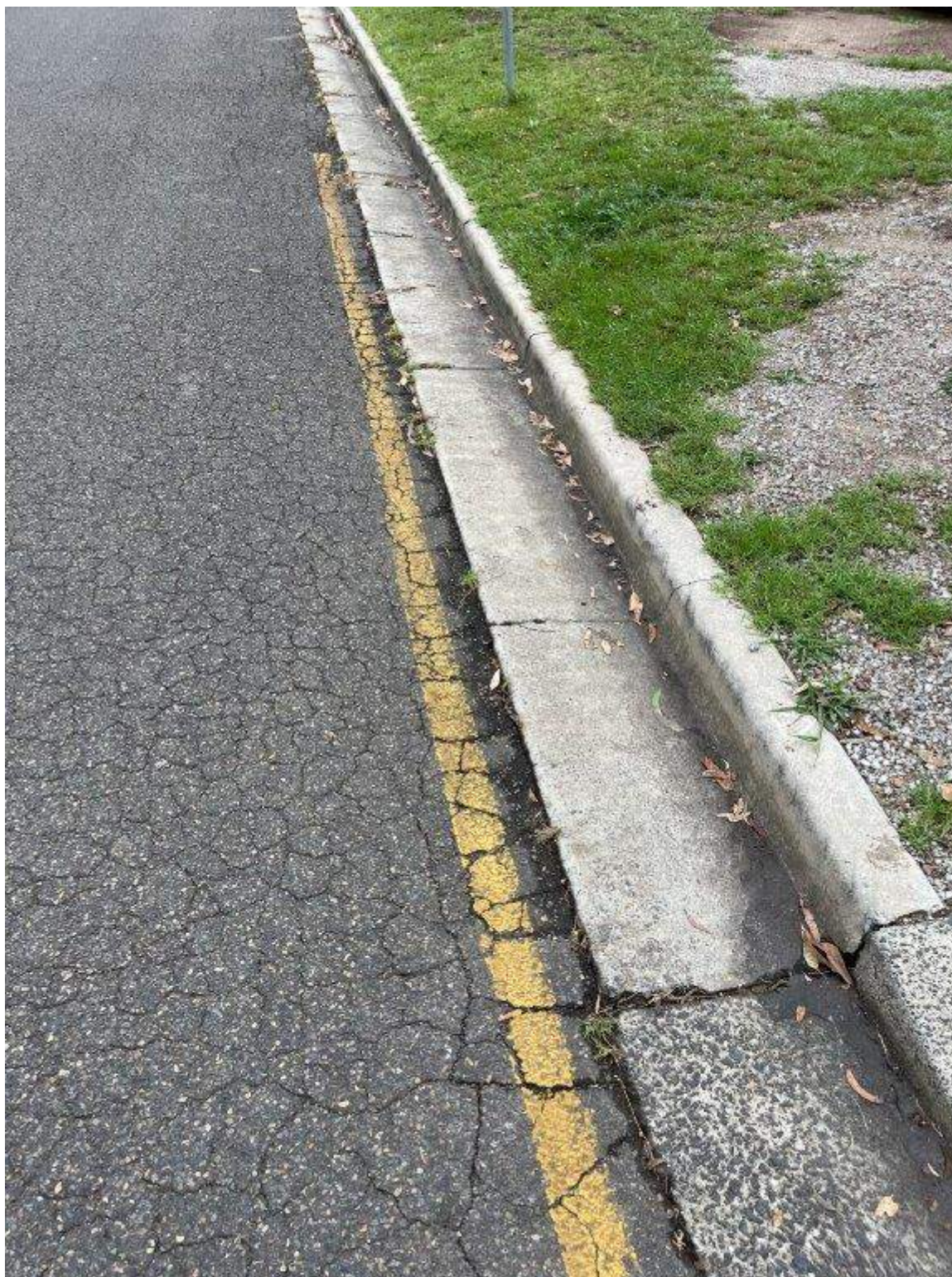
Photo 206 - Taren Point Road - Cracking of pavement
