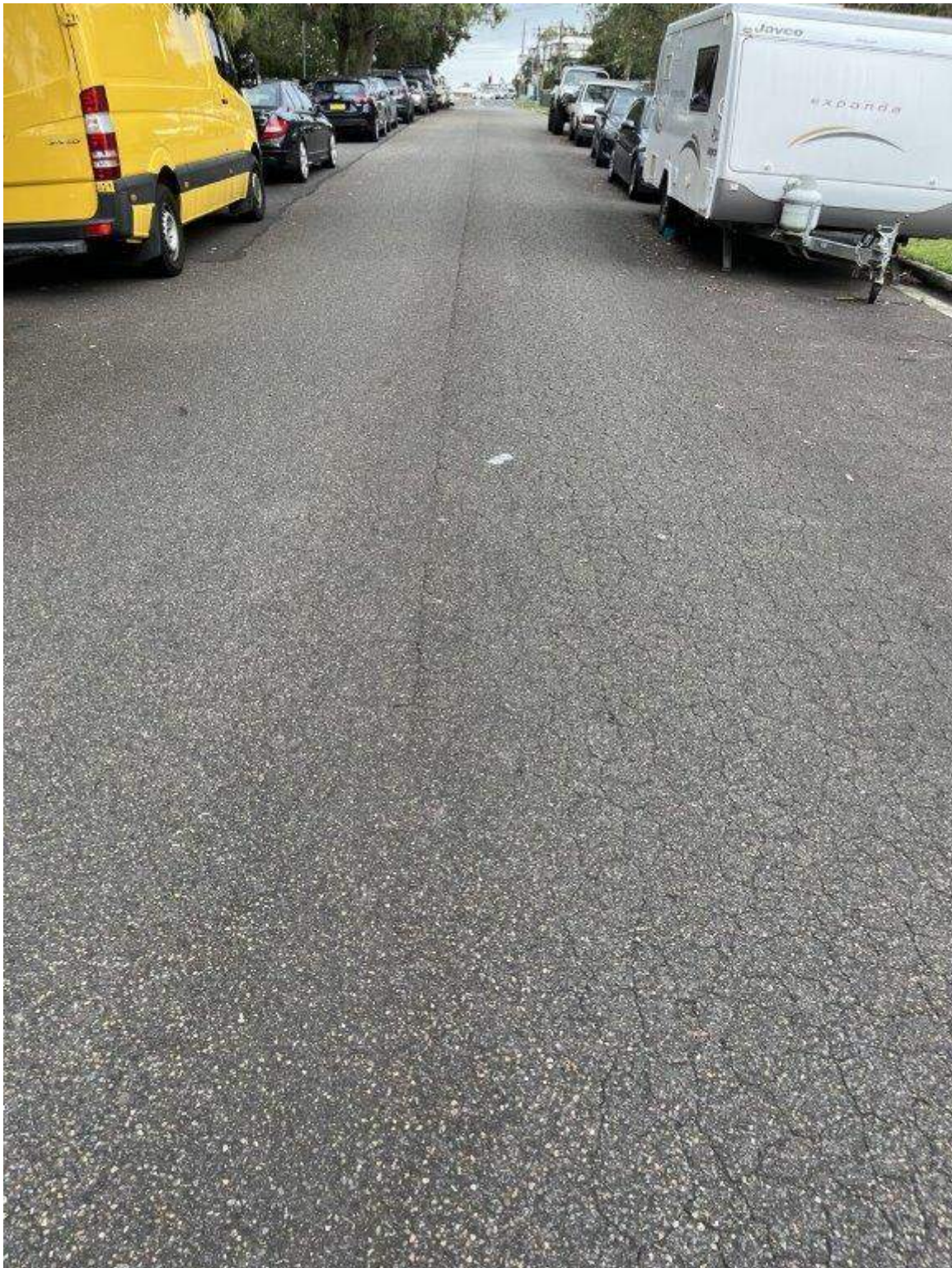
Photo 168 - Taren Point Road - Cracking of pavement
