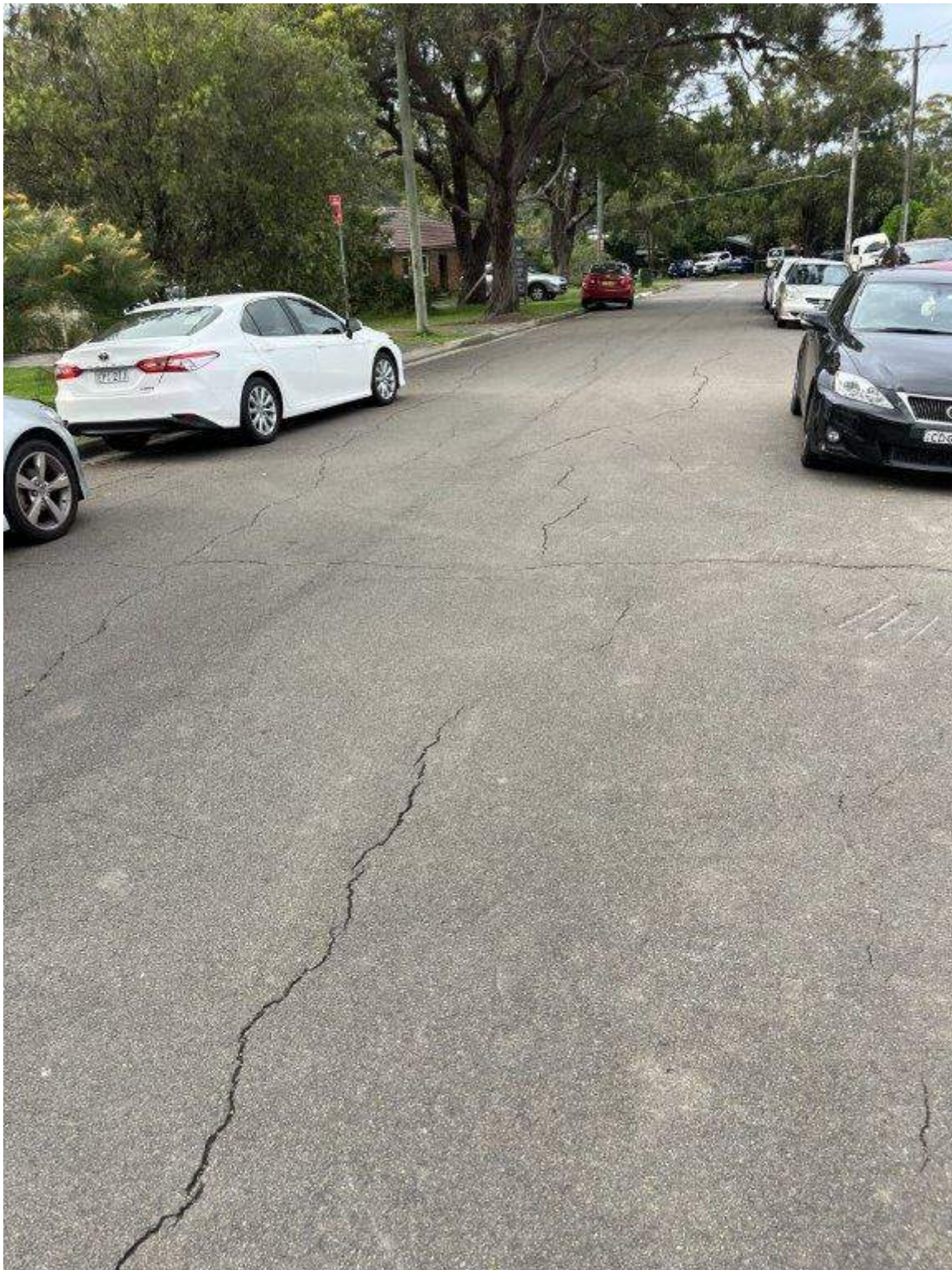
Photo 76 - Hinkler Avenue - Cracking of pavement
