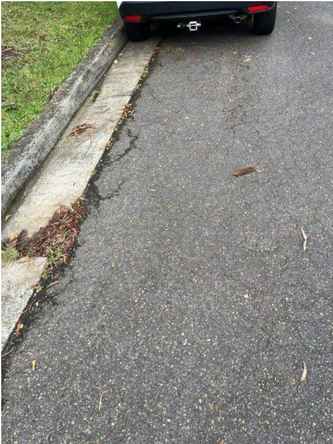
Photo 163 - Taren Point Road - Cracking of pavement
