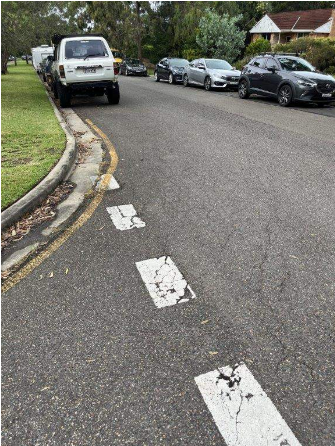
Photo 192 - Taren Point Road - Cracking of pavement
