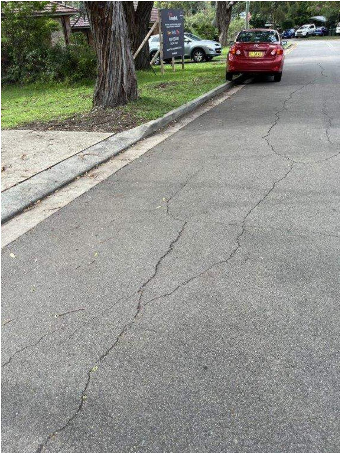
Photo 91 - Hinkler Avenue - Cracking of pavement
