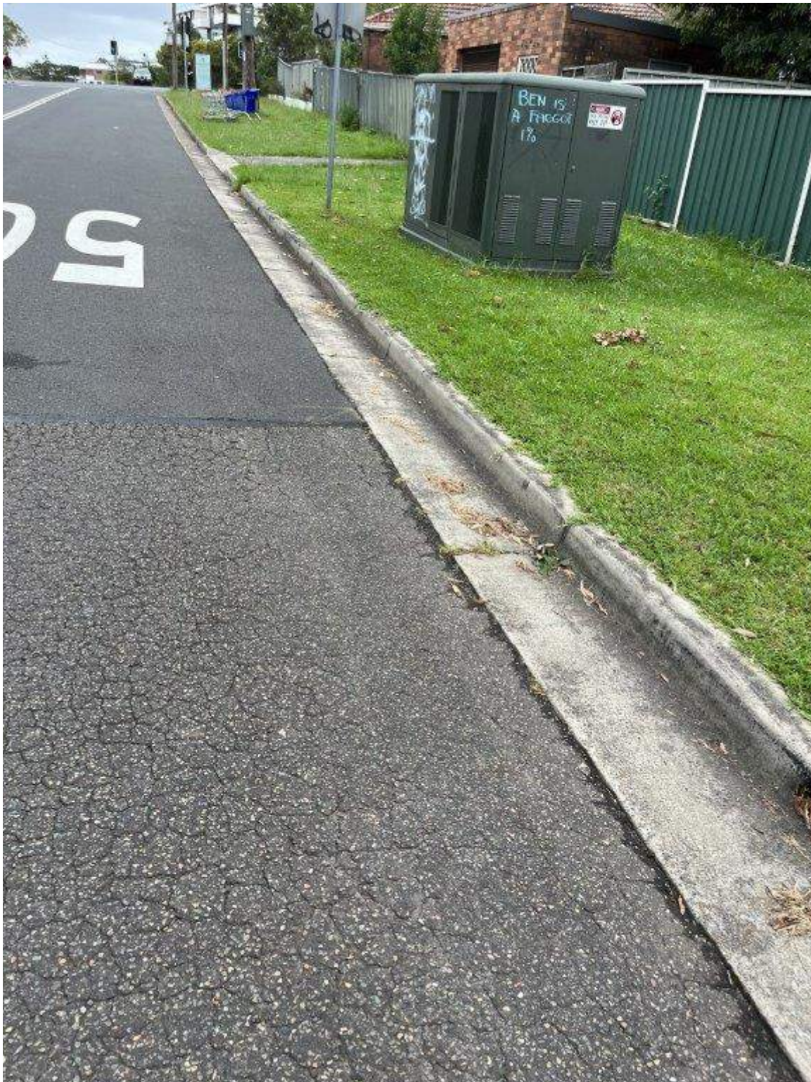
Photo 222 - Taren Point Road - Cracking of pavement
