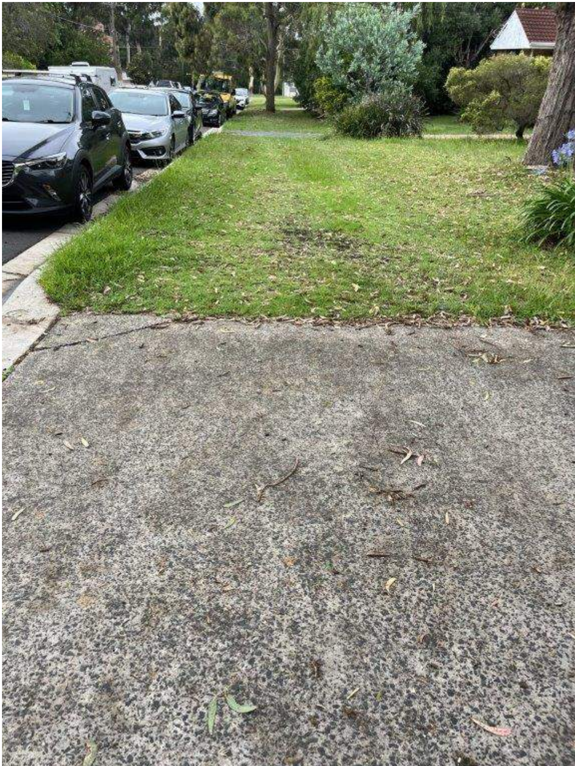
Photo 195 - Taren Point Road - Cracking of pavement
