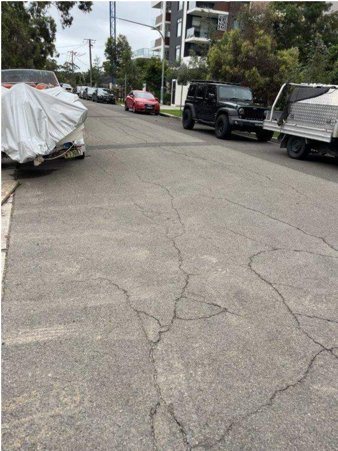
Photo 29 - Hinkler Avenue - Cracking of pavement
