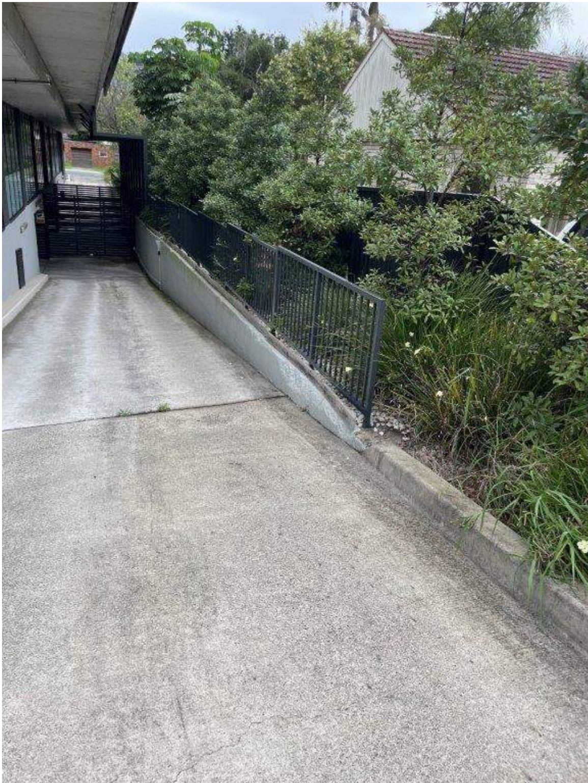
Photo 25 - Hinkler Avenue - Cracking of pavement
