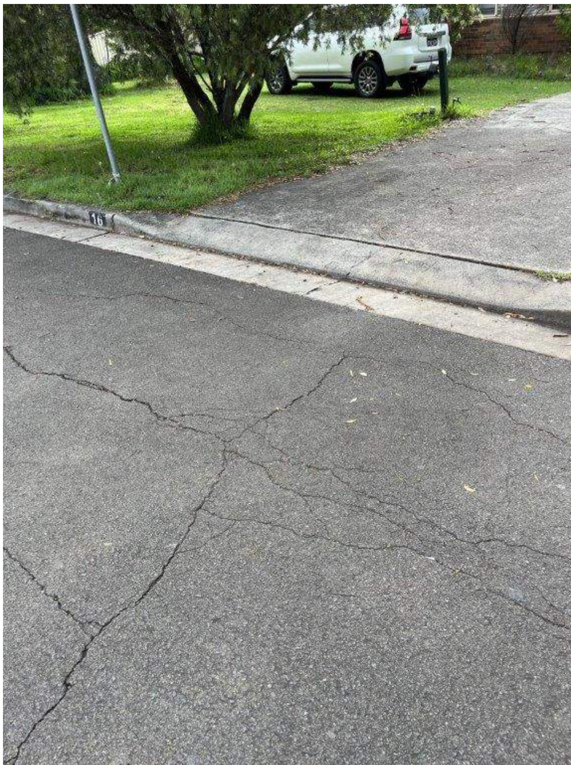
Photo 89 - Hinkler Avenue - Cracking of pavement
