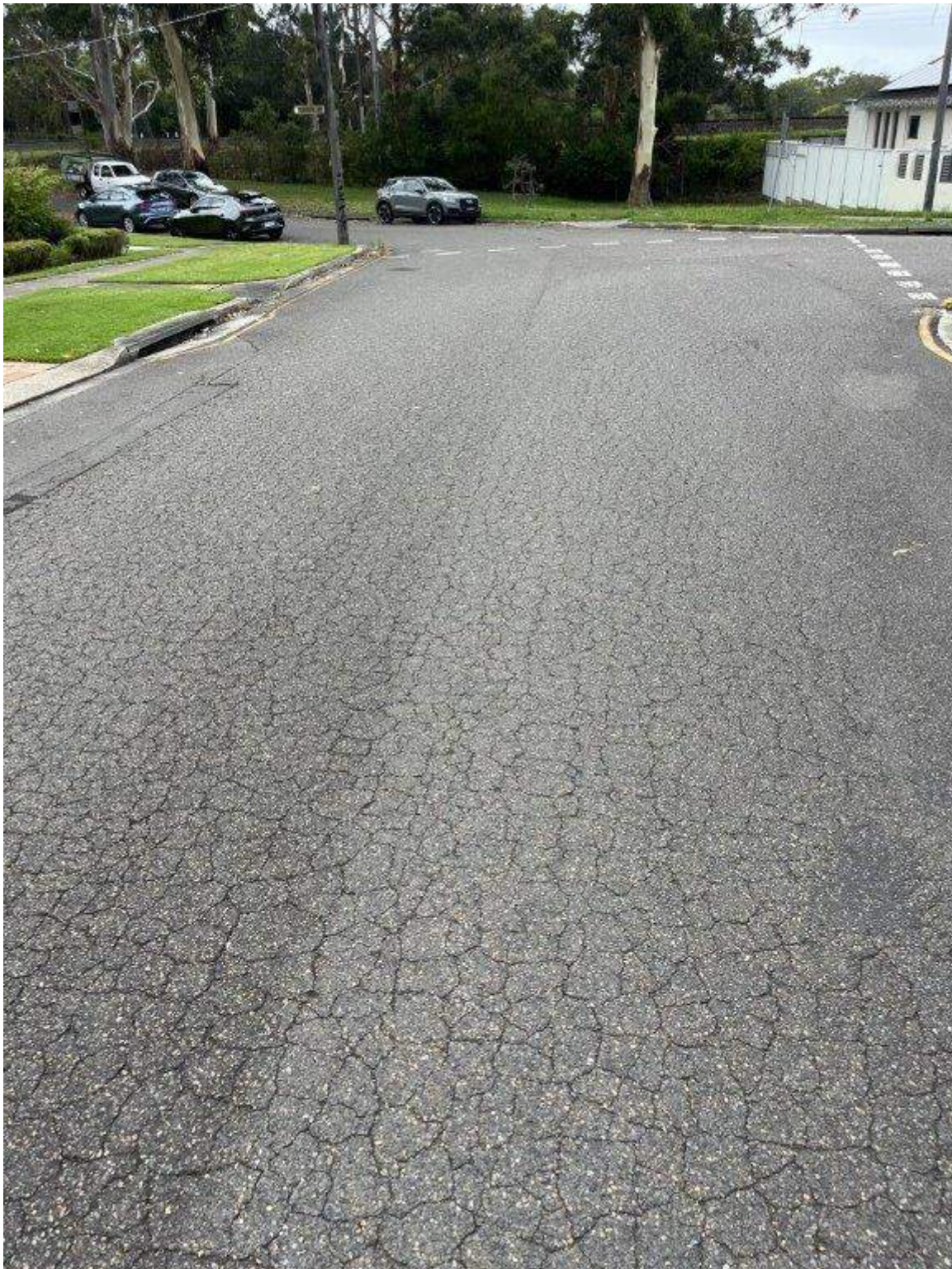
Photo 152 - Taren Point Road - Cracking of pavement
