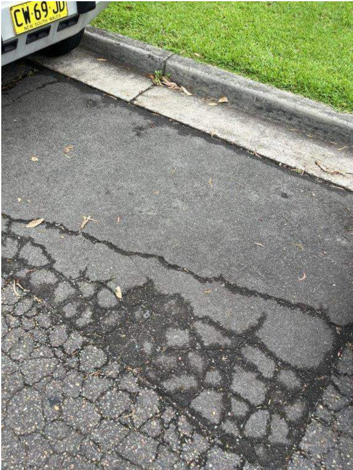
Photo 154 - Taren Point Road - Cracking of pavement
