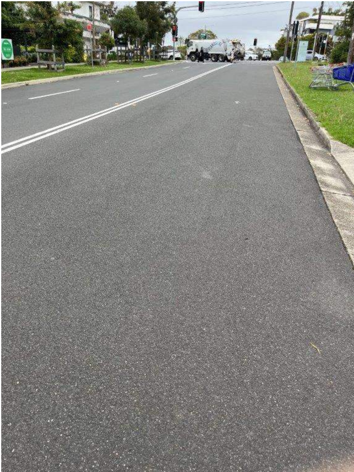
Photo 227 - Taren Point Road - Existing condition of pavement
