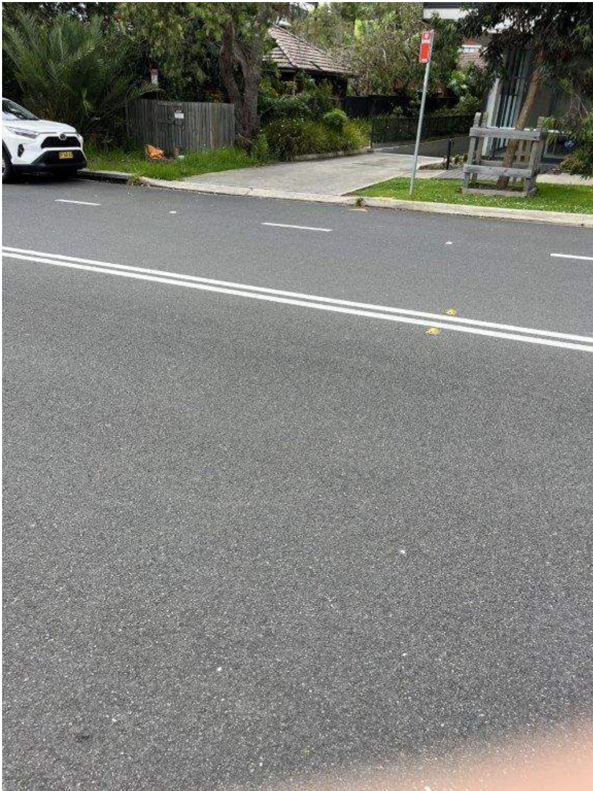
Photo 235 - Taren Point Road - Existing condition of pavement
