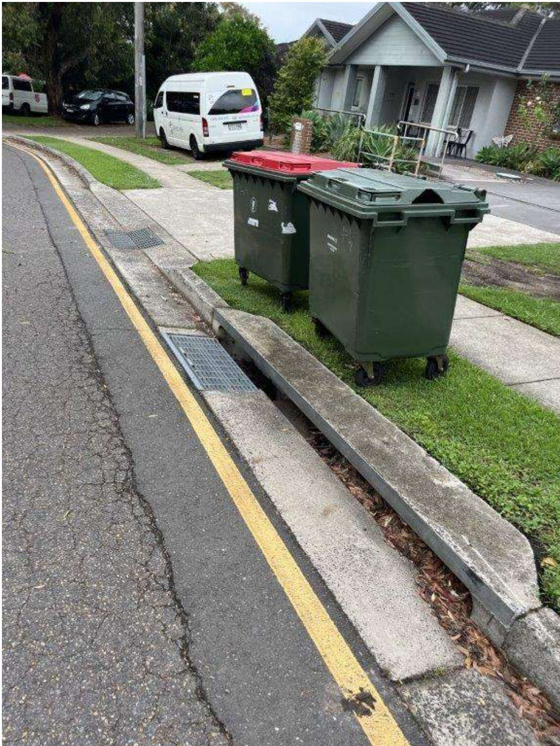
Photo 105 - Hinkler Avenue - Cracking of pavement
