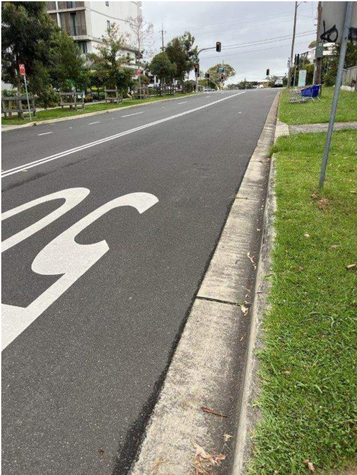
Photo 224 - Taren Point Road - Existing condition of pavement
