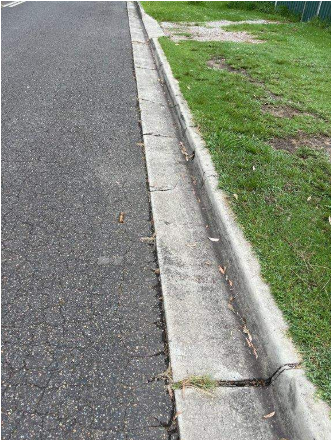
Photo 215 - Taren Point Road - Cracking of kerb and pavement
