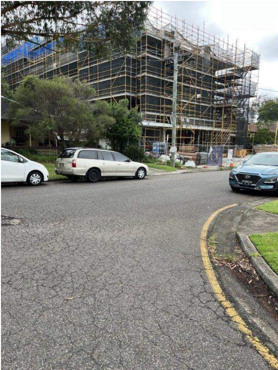
Photo 188 - Taren Point Road - Cracking of pavement
