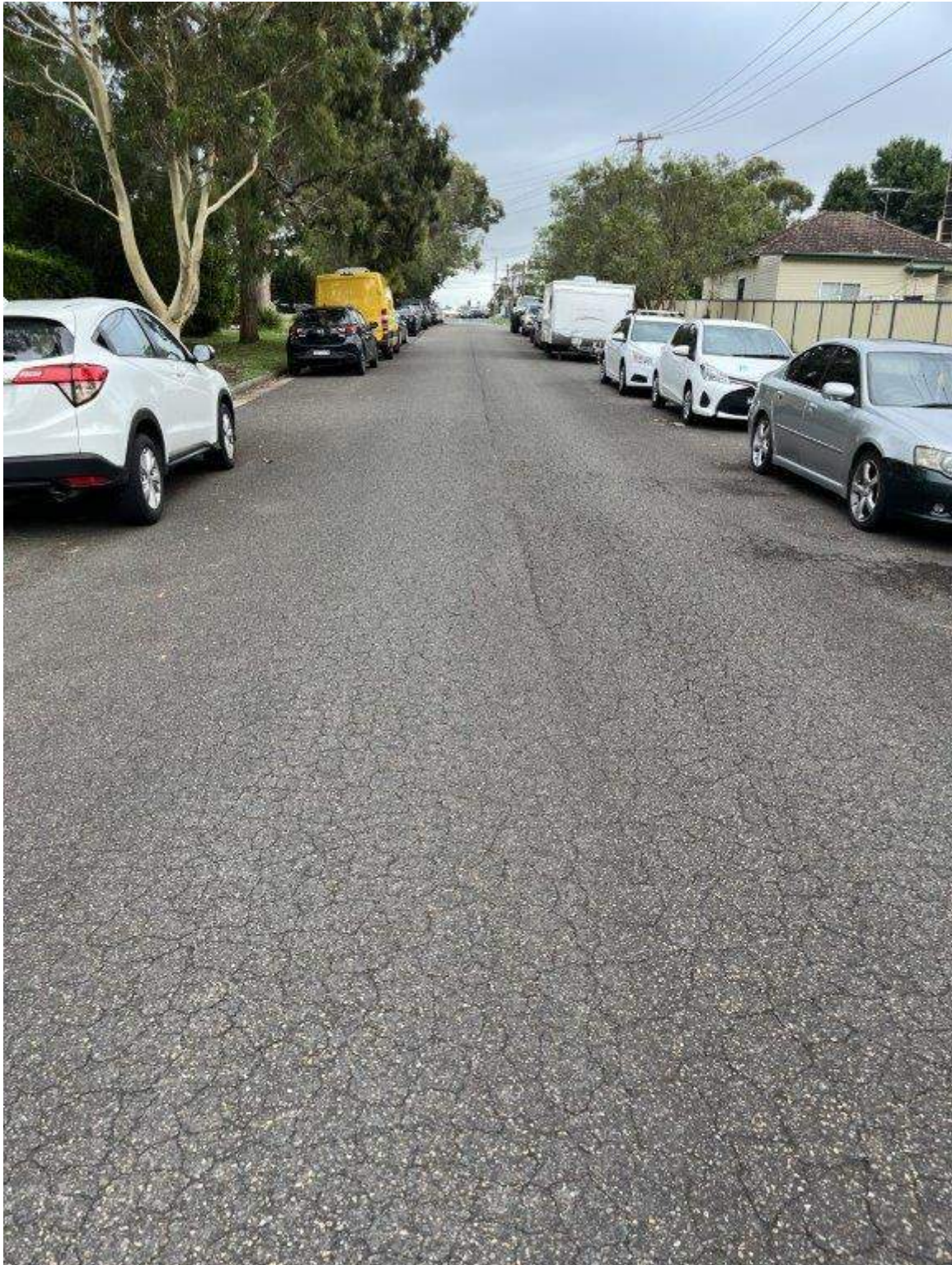
Photo 160 - Taren Point Road - Cracking of pavement
