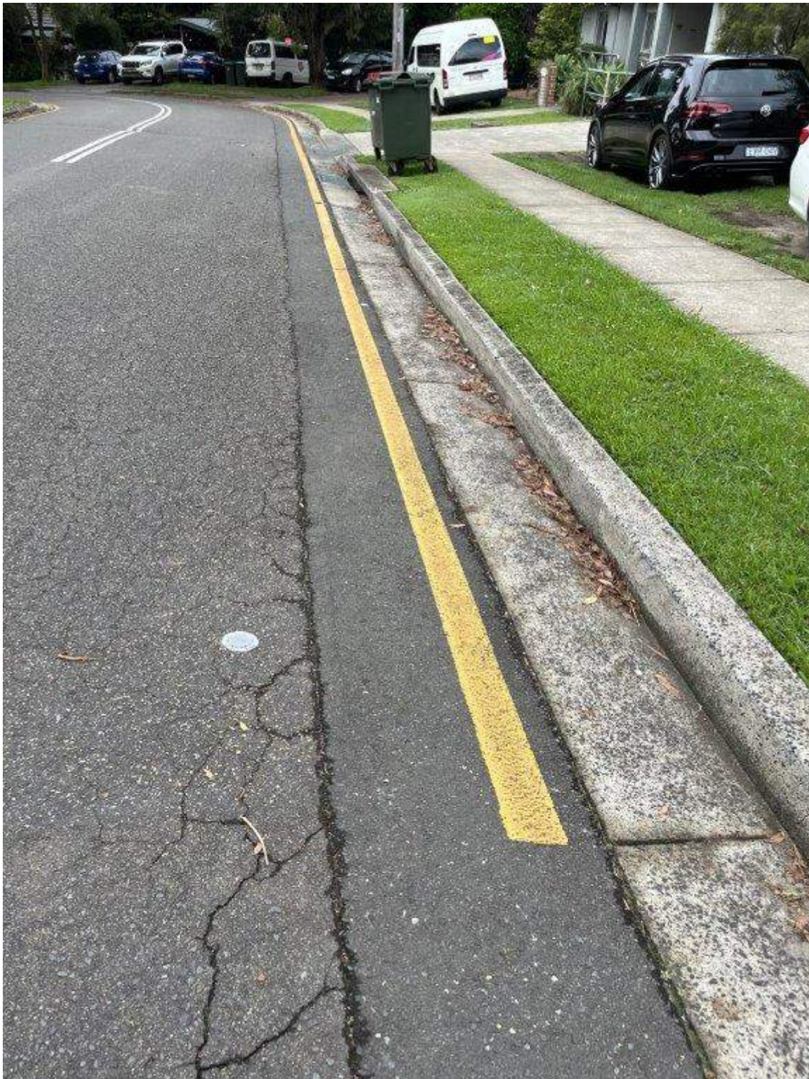
Photo 102 - Hinkler Avenue - Cracking of pavement
