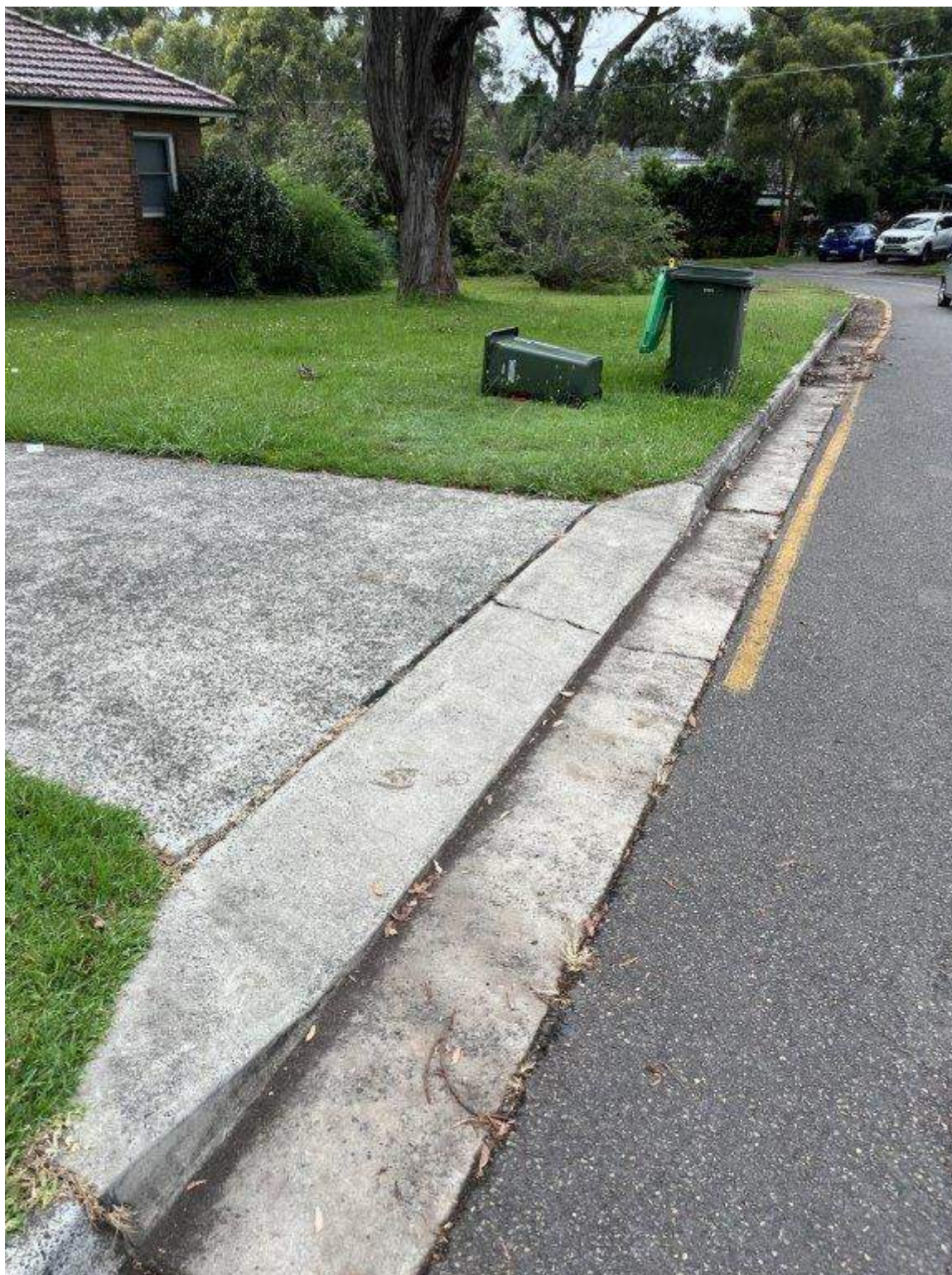
Photo 104 - Hinkler Avenue - Cracking of pavement
