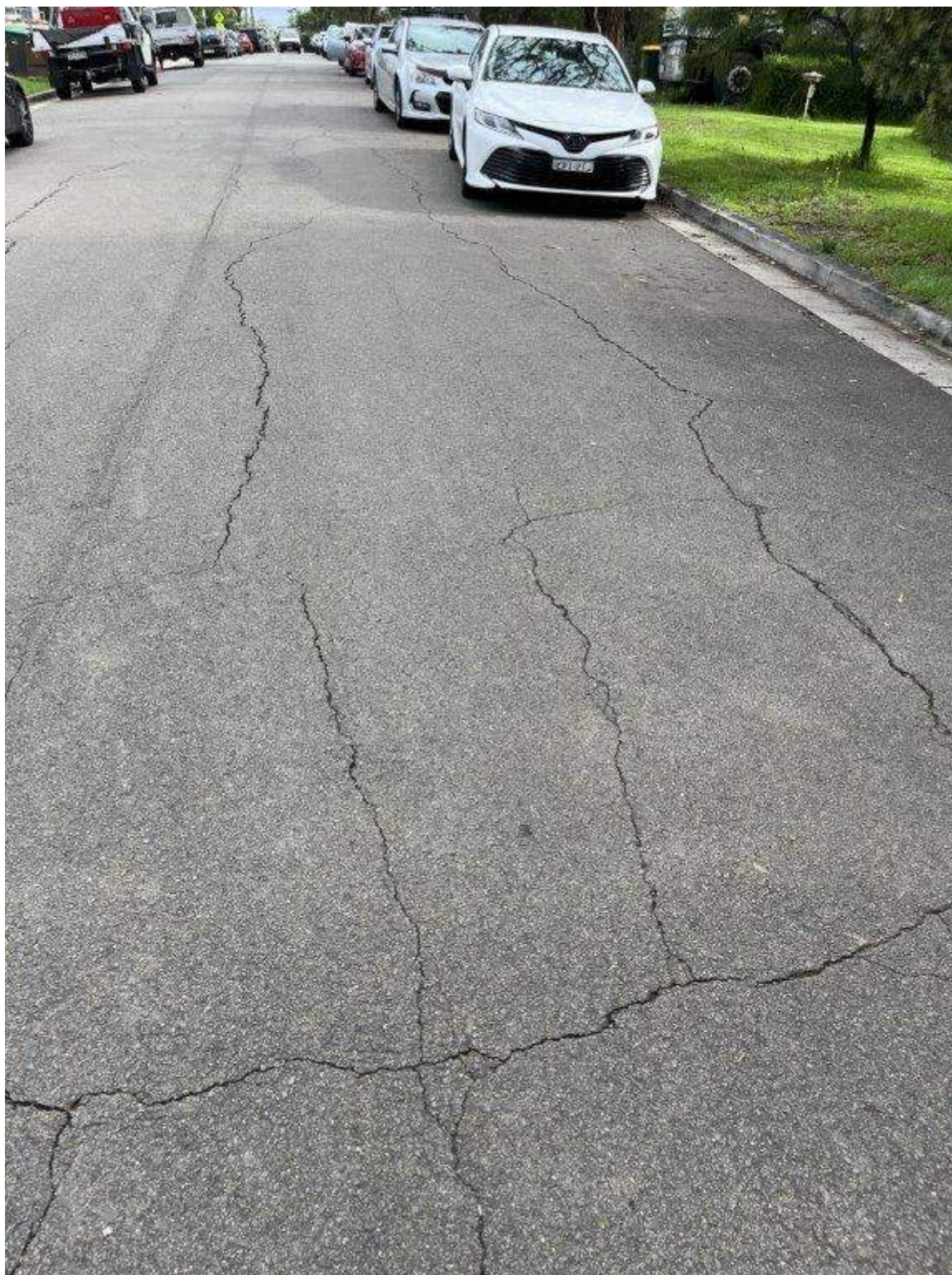
Photo 90 - Hinkler Avenue - Cracking of pavement
