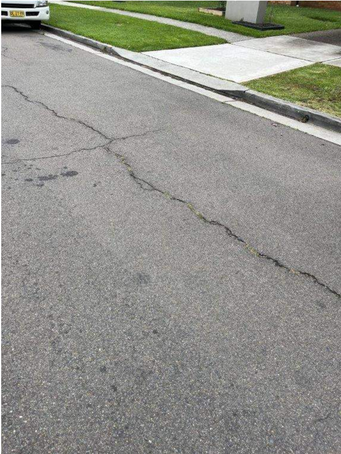
Photo 17 - Hinkler Avenue - Cracking of pavement
