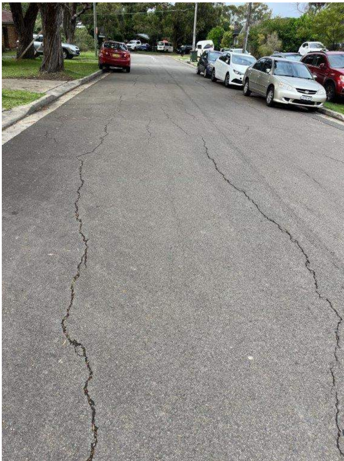
Photo 85 - Hinkler Avenue - Cracking of pavement
