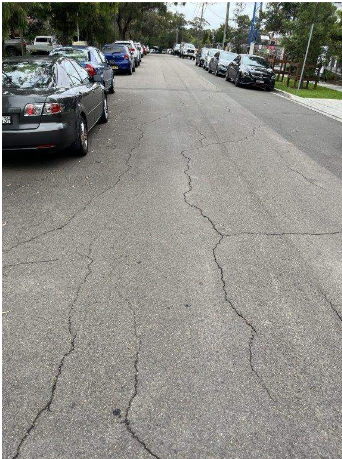
Photo 33 - Hinkler Avenue - Cracking of pavement
