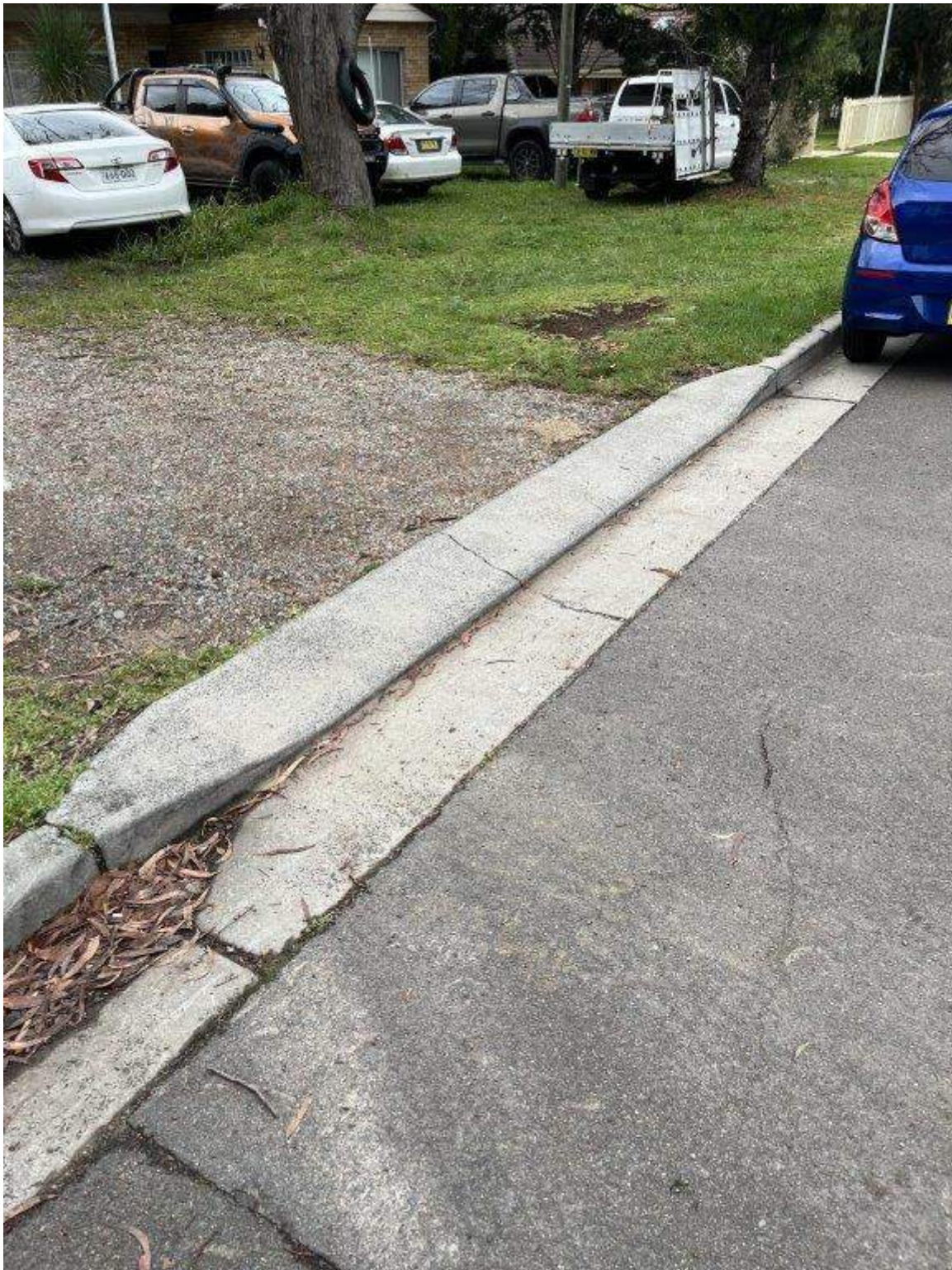
Photo 51 - Hinkler Avenue - Cracking of pavement
