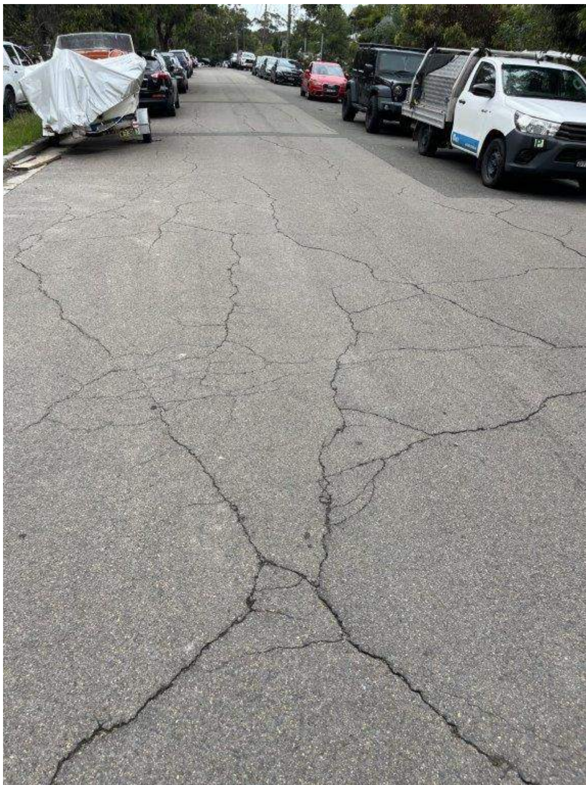
Photo 20 - Hinkler Avenue - Cracking of pavement
