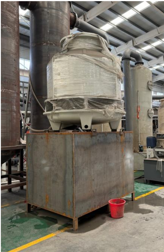
Figure 6-21 Single fan water cooling tower unit installed internally on LIB recycling equipment during the factory acceptance test at the OEM site
