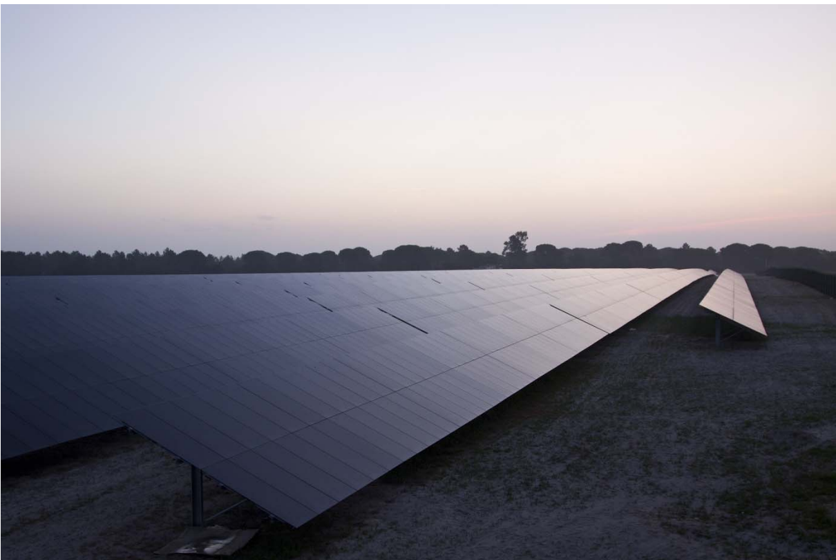
Figure 1-4 2.2MWp solar project constructed in Coruche, Portugal (Source Neoen Australia, 2014)
