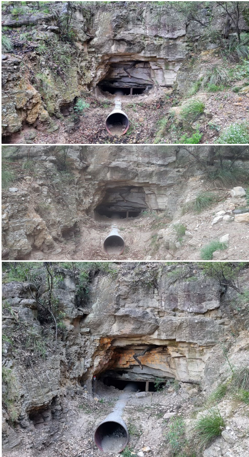
Plate 5-1: Periodic monitoring photo of adit entrance from February 2021 (top), January 2022 (middle) and December 2022 (bottom) showing lack of substantial change
