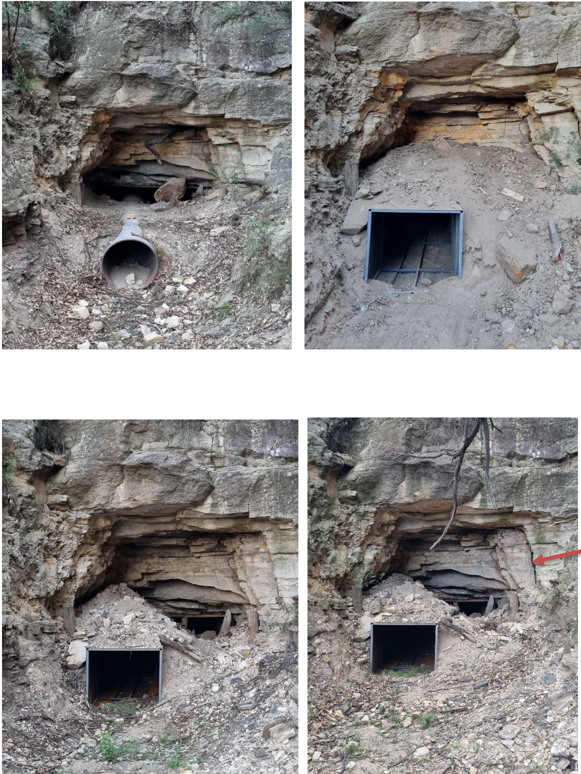
Plate 5-2: Monitoring photos of adit entrance pre culvert installation (March 2023 – top left), afternoon of installation (April 2023 – top right), nine months after installation (January 2024 – bottom left), and 20 months after installation (December 2024 – bottom right). This shows progression of pipe to tunnel with
