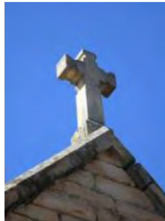
Plate 62. Evidence of re-mortaring between the sandstone blocks.
