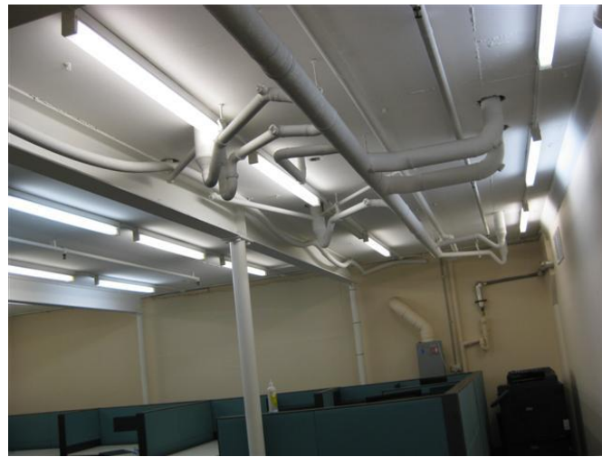
PLUMBING IN CELING OF ROOM G.16
