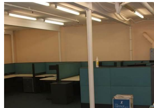
View of room G16 with steel framing and reinforced concrete mezzanine floor slab
