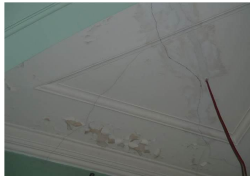
Room 316 cracking to corner transition to dome
