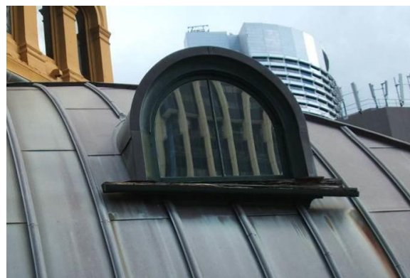
Split and rotted sill loose and dislodged
