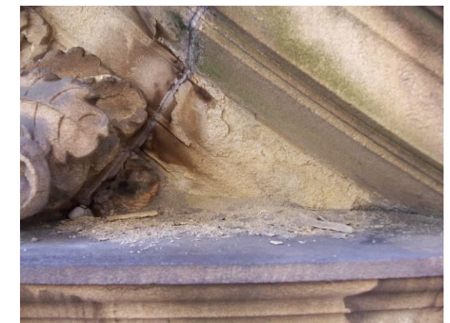
Salt contamination and damage to Loftus Street entrance carvings
