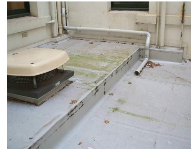
Membrane roof over room G28 cleaning required
