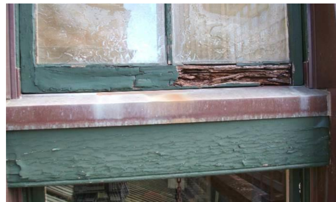
Rot in dome window sash
