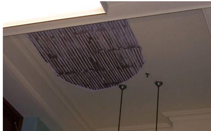
Lath and plaster ceiling failure in 2007
