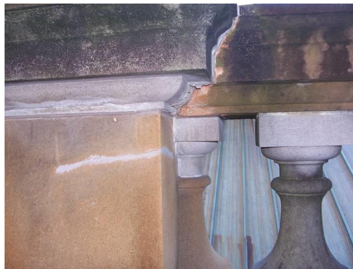
Parapet cracking, past stone replacement
