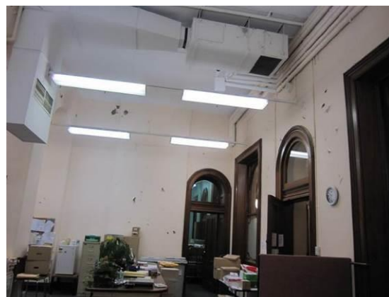
Ground floor office, services within room
