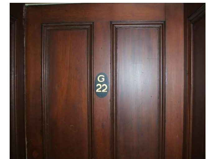
Typical four panel door with gilt door numbering Room G 22 (Ground floor)
