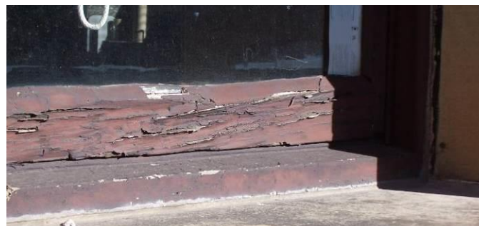
Bottom rail rot & failing paint
