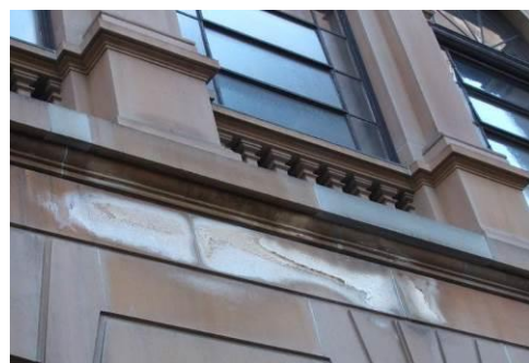
Salt damp damage outside rooms 107A & B
