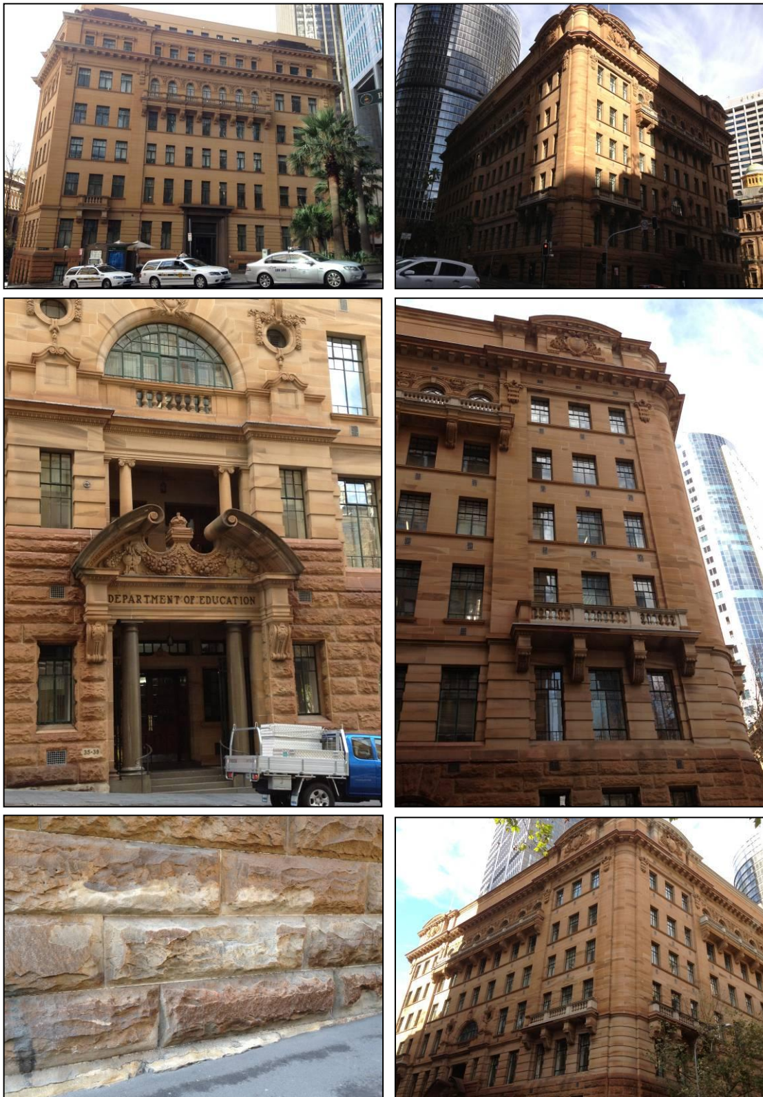
Figure 4.5: External views of the Department of Education Building. Clockwise from top left: Farrer Place facade, corner Bridge & Young Streets, detail of northernmost bay of Young Street facade, view from the corner Bridge & Loftus Streets, an example of exfoliation on the base rusticated stonework on Farrer Place facade, and Bridge Street entrance portico
